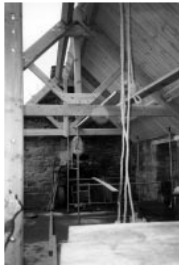
Bothy renovation at Wester Lawrenceton by Edge Architecture and Design. New roof structure of local douglas fir - breathing roof insulated with "Warmcel" - (blown cellulose insulation made from re-cycled newsprint).
