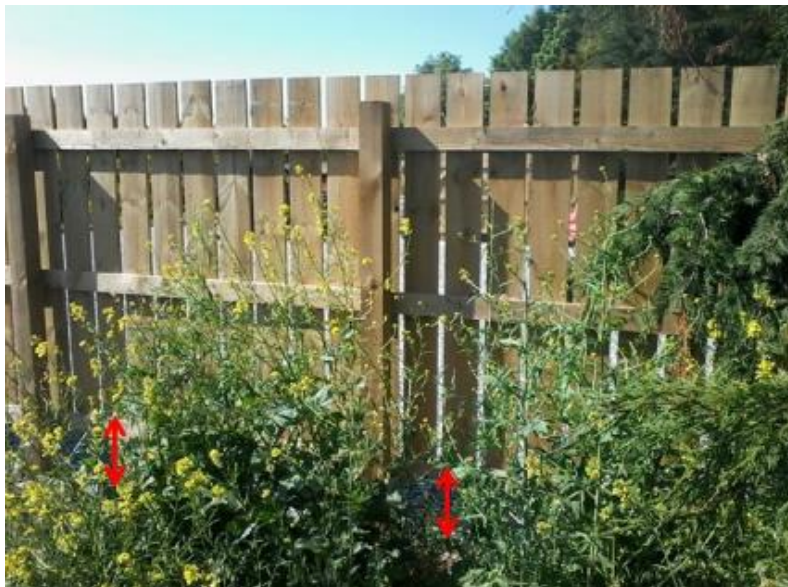
Plate 1: Gap at bottom of fencing as a result of the removal of the lower section
