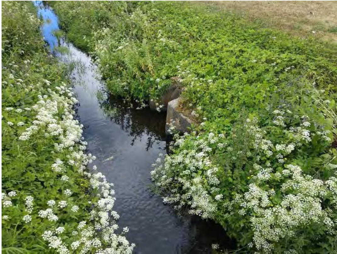
Photography 13. Surface water discharge between Section SX14 and Section SX15.
