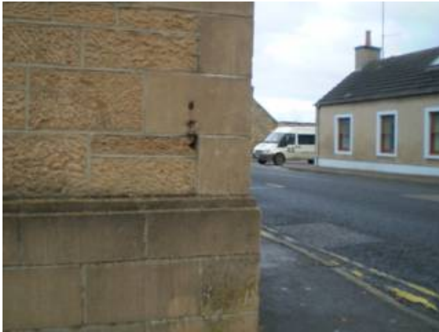
Available visibility to north of access at 2.4 metres, from the edge of the carriageway.
