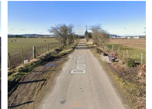
4c - condition of road
