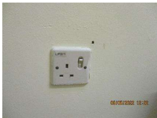
191. Electrical power – socket / dining block example.
