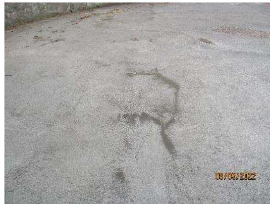
203. Evidence of water ponding
