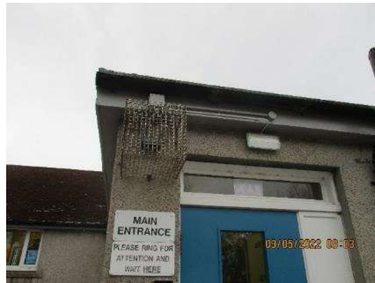
159. External lighting – teaching block.
