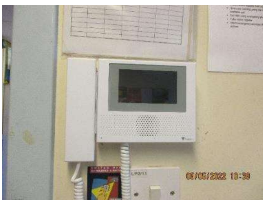
171. Door access system receiver handset and viewer. Reception office - teaching block.
