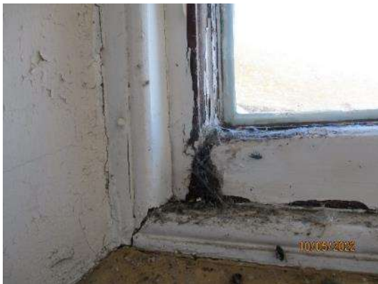
63. Wet rot in sashes and frames
