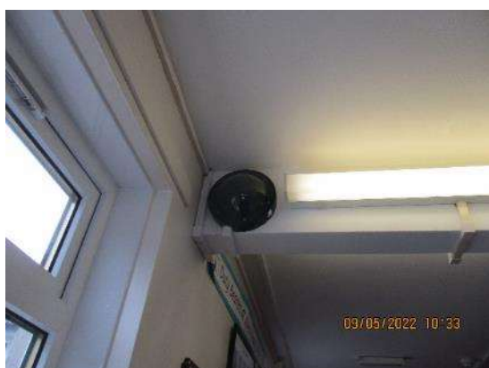
172. CCTV camera – main entrance / teaching block.
