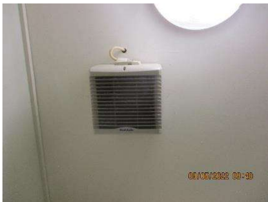
144. Extract fan – teaching block toilet.
