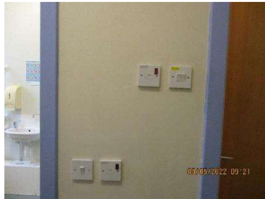
153. Electrical power – isolation switches teaching block toilets.
