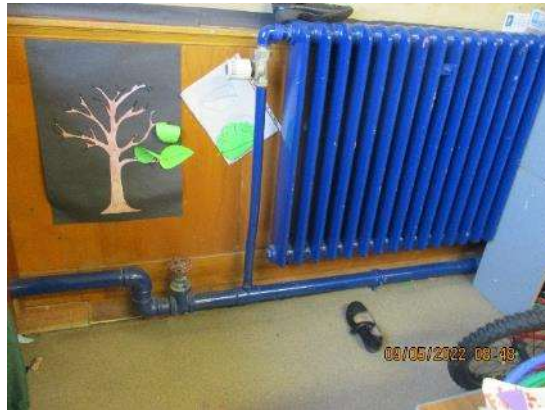
137. Radiator – heating system teaching block example.
