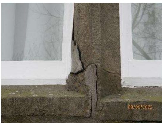
65. Damage/repairs to stone mullions
