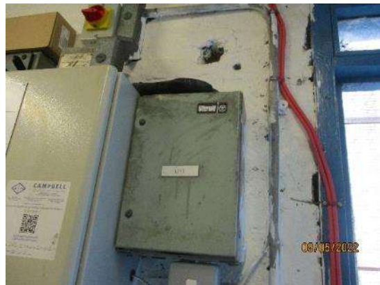
189. Electrical power – distribution board. Dining block.
