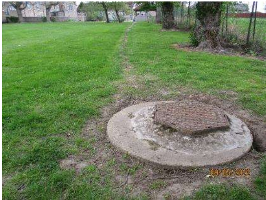
220. Raised manhole covers
