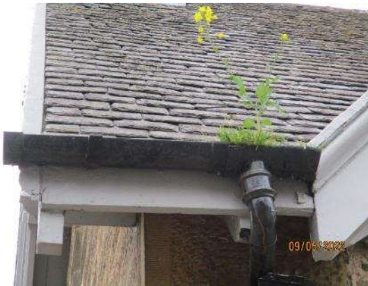
31. Vegetation in rainwater goods
