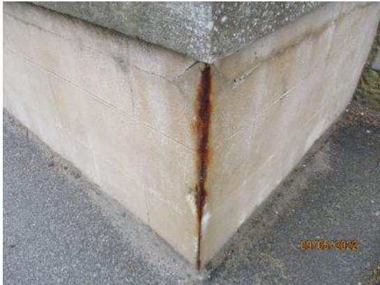
78. Corcor bead corrosion
