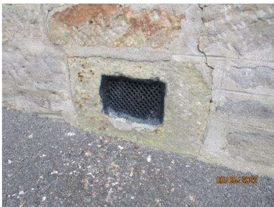
47. Below floor ventilation – Dining block
