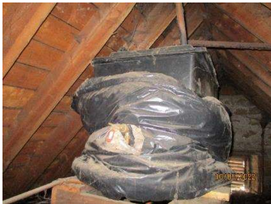
176. Heating feed and expansion tank. Dining block attic.
