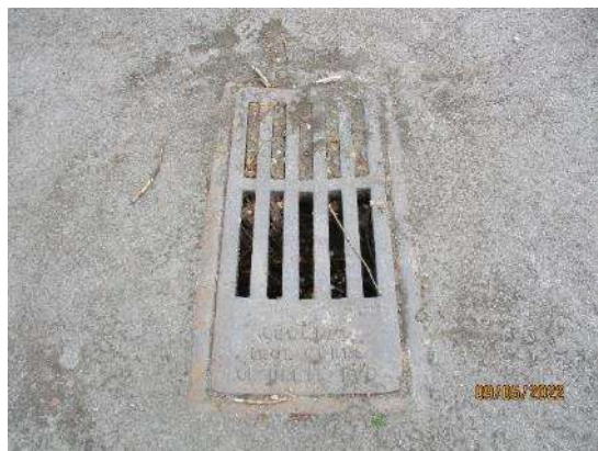
217. Road gullies, part blocked
