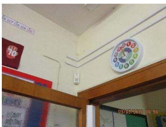
169. Intruder alarm system detector - teaching block.
