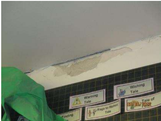
103. Plastered walls - spalling
