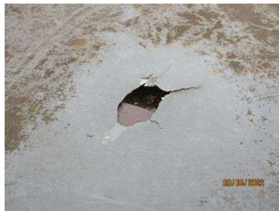
18. Hole in GRP roof
