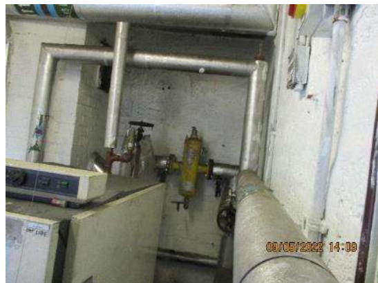
179. Heating pipework and valves. Dining block.
