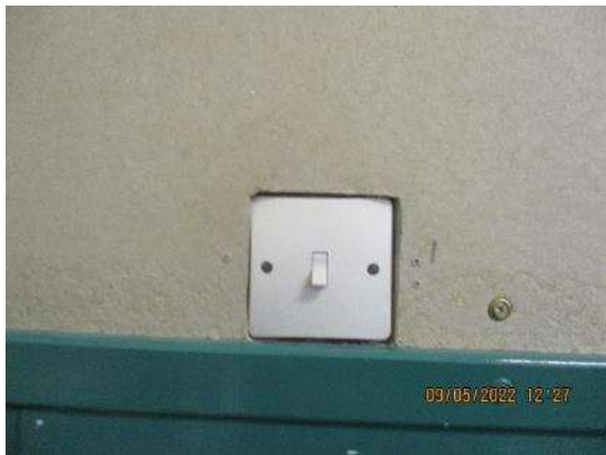
194. Light switch – dining block gym store.
