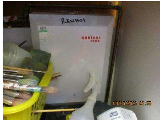
141. Point of use electric water heater. Teaching block classroom typical.
