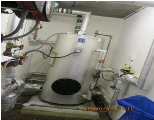
180. Hot water calorifier – dining block boilerhouse.
