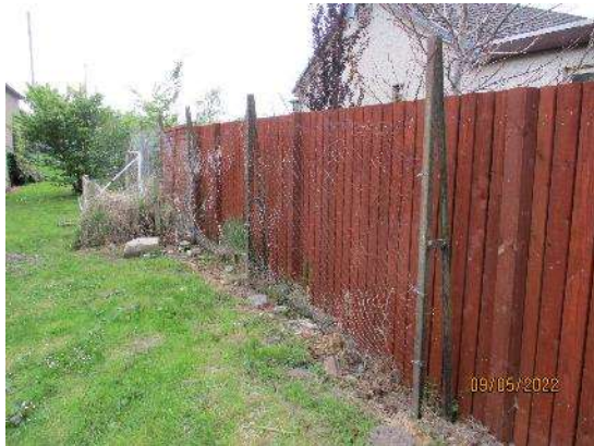
208. Damaged chain link fencing
