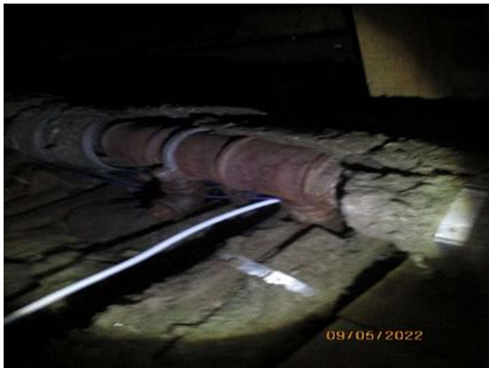
136. Pipework – Heating system distribution in teaching block attic.
