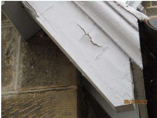
27. Wet rot to rafter feet
