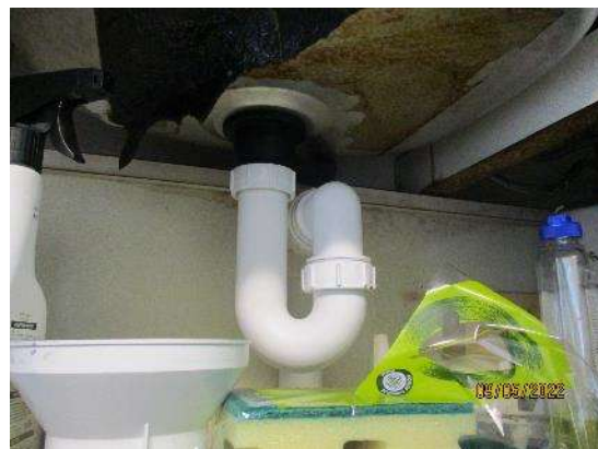
129. PVC waste pipes
