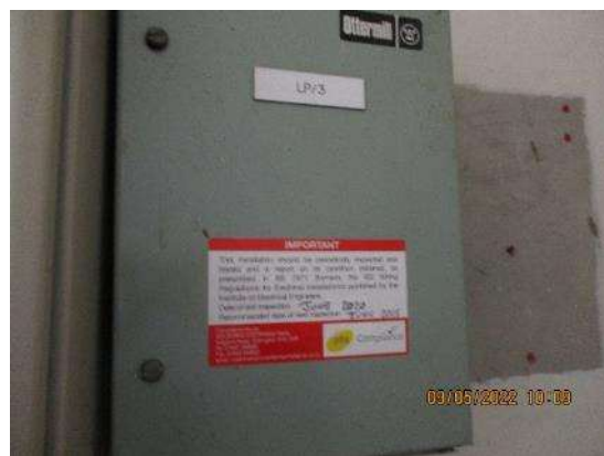
151. Electrical power distribution board – teaching block
