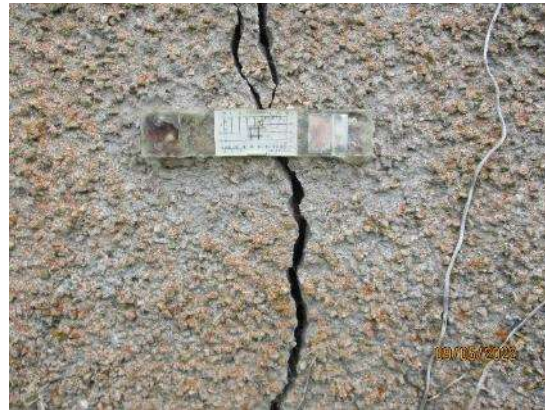
40. Extensive, significant cracking
