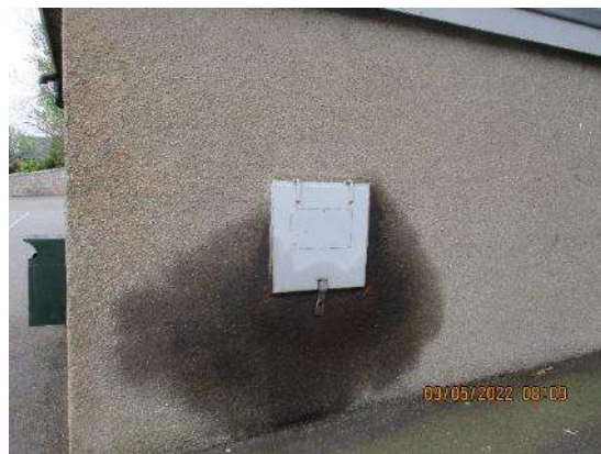
185. Oil tank fill point – dining block.
