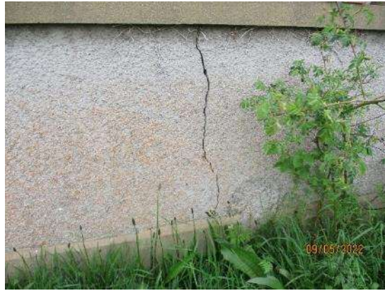
50. Cracked roughcast – Teaching north
