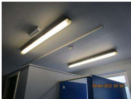
156. Lighting – teaching block boys toilets.
