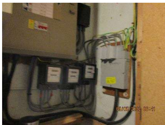
150. Incoming power supply/meters/fuses teaching block
