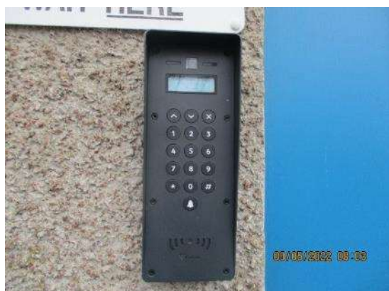
170. Door access system control keypad main entrance. - Teaching block.
