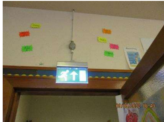
161. Emergency exit sign light. Teaching block.
