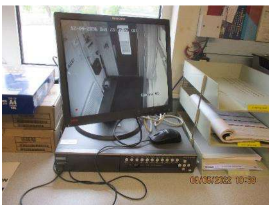
173. CCTV system monitor and recorder. Teaching block reception office.
