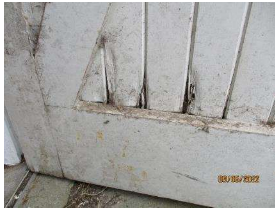
56. Wet rot in lining boards
