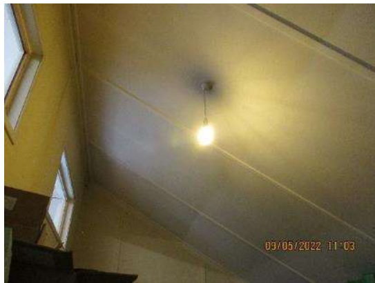
195. Lighting – dining block store.
