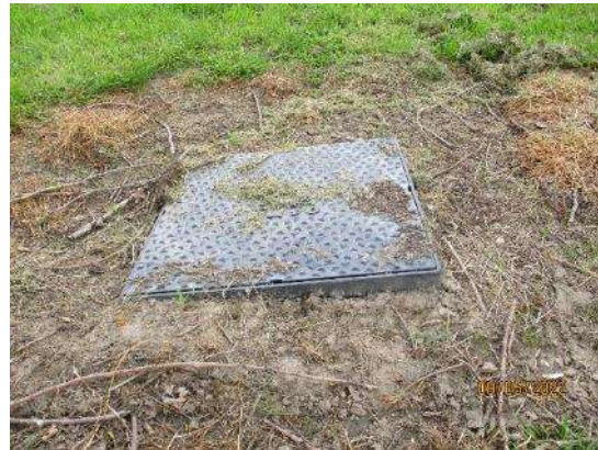
221. Insecure manhole covers
