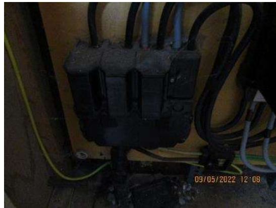
187. Incoming power supply and main fuses dining block.
