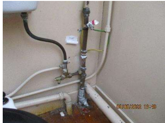
143. Cold water copper pipework – teaching block typical.
