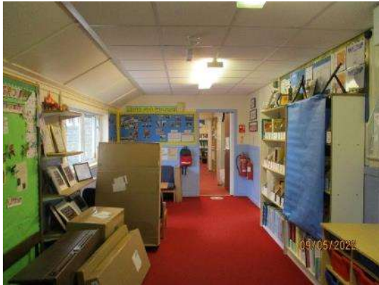
95. Suspended ceiling tiles
