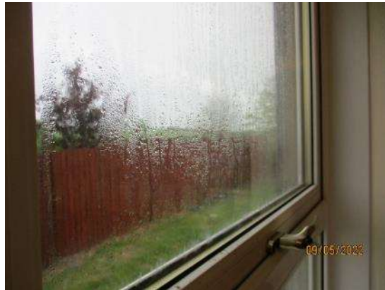
70. Failed double glazed units
