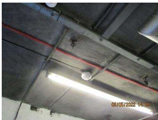
197. Fire alarm system. Wiring and detector head. Dining block.
