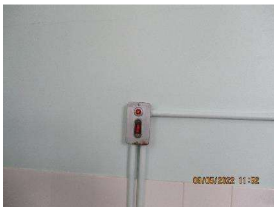
190. Electrical power – Isolation switch – dining block kitchen.
