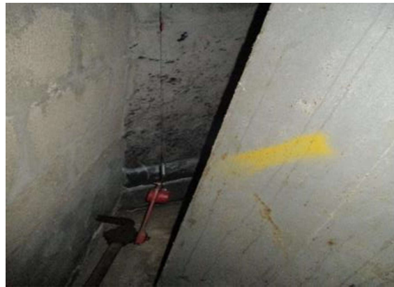
147. Oil supply automatic shut off valve – teaching block.
