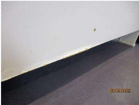
127. Water damage to bottom edge
