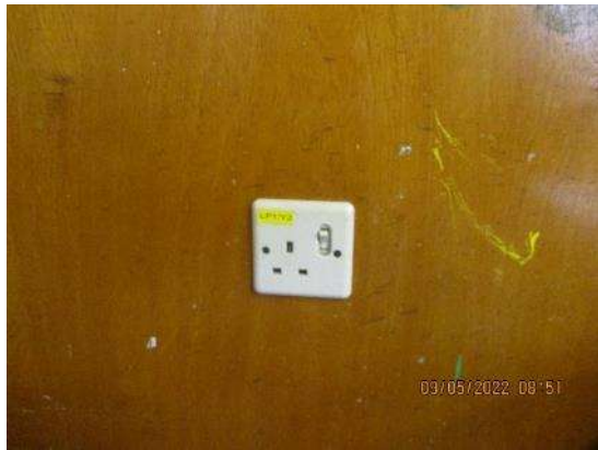
152. Electrical power – socket teaching block example.
