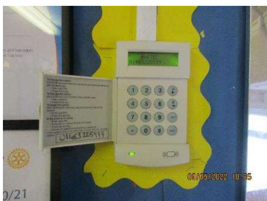
168. Intruder alarm keypad – teaching block entrance lobby.
