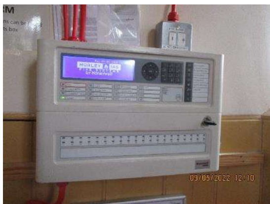
196. Fire alarm control panel. Dining block 1/20.
