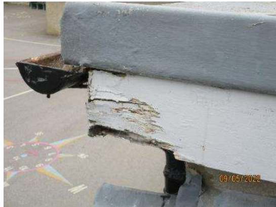
28. Wet rot to fascia boards
