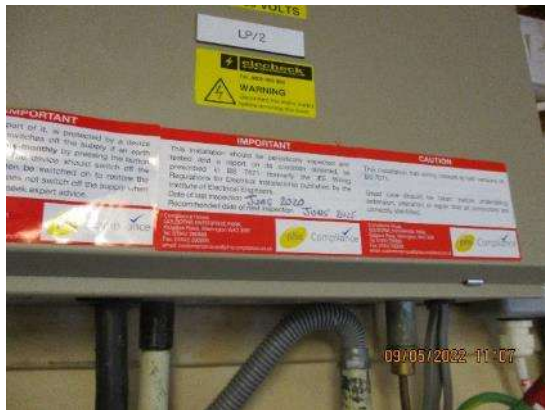
148. Electrical power – distribution board – teaching block.
