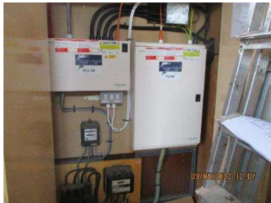
188. Electrical power distribution boards. Dining block.
