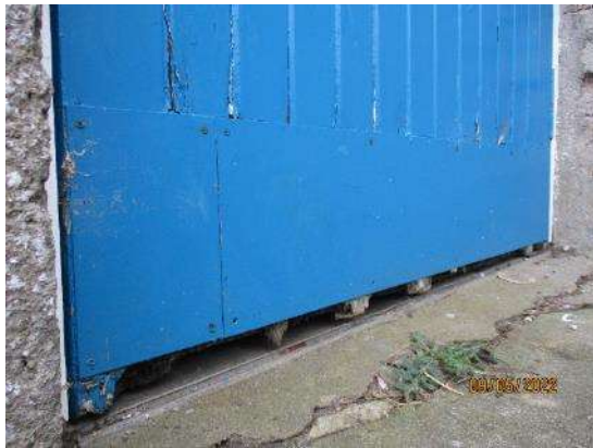
55. Wet rot in bottom rail
