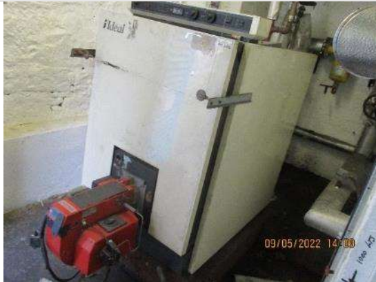
174. Oil fired boiler. Heating and hot water.
