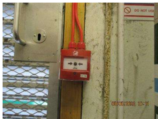
163. Fire alarm device. Call point – teaching block.
