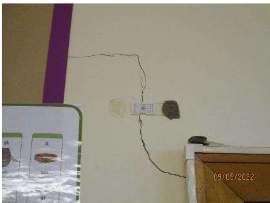
105. Plastered walls - cracked
