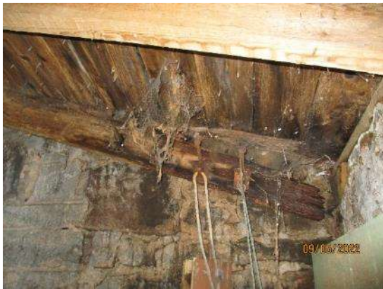
7. Lean-to store – extensive wet rot
