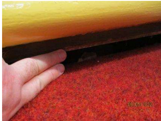
81. Concrete floor subsided
