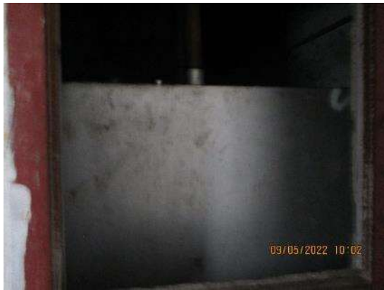
146. Oil tank in bunded store – teaching block.
