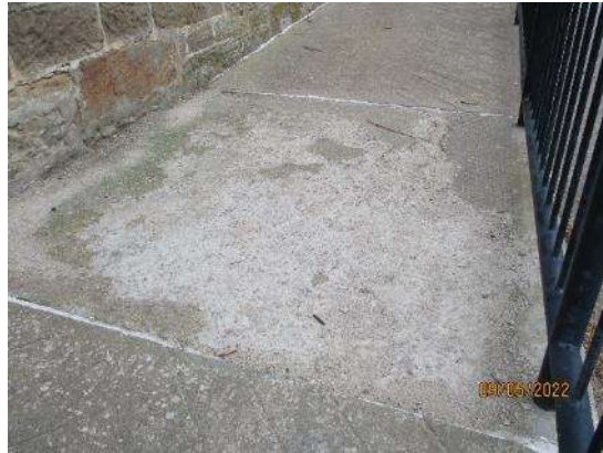
79. Eroded concrete surface
