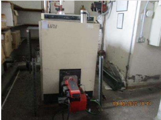
134. Oil fired heating only boiler.
