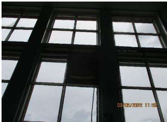
186. Extract fan – dining block kitchen window.
