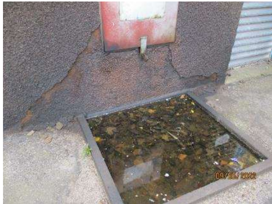
51. Damaged roughcast – Plant room
