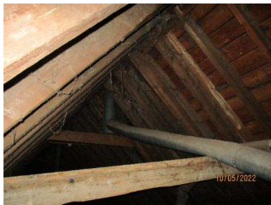
6. Dining block – vent pipes resting on structure
