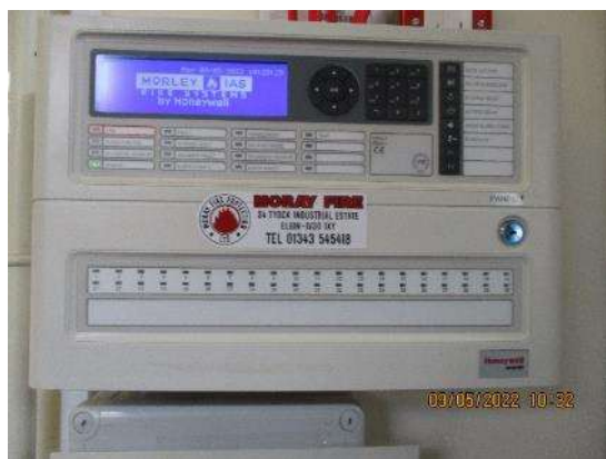
162. Fire alarm control panel. Teaching block entrance.
