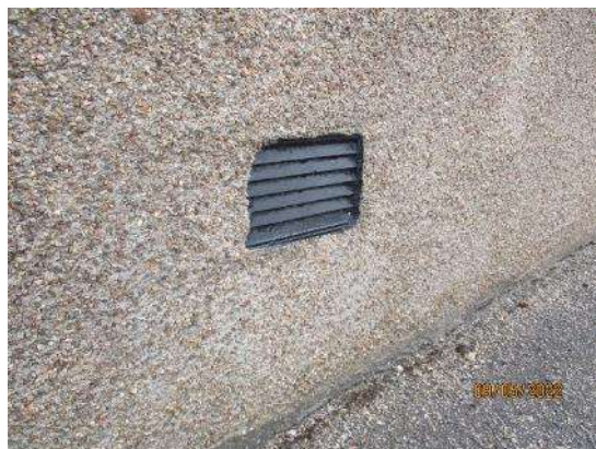
48. Below floor ventilation – Teaching south
