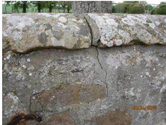
215. Cracks and movement adjacent to trees
