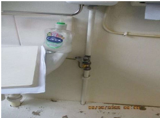
142. Cold water copper pipework – teaching block typical
