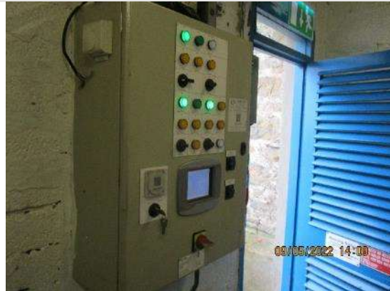
175. Heating BEMS control panel dining block boilerhouse.
