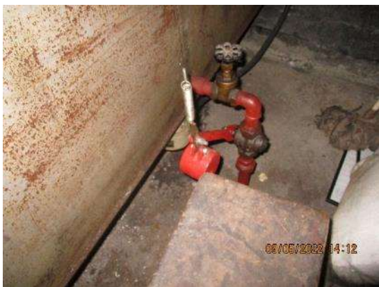
184. Oil control safety shut off valve. Dining block.
