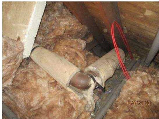
177. Heating pipework. Dining block attic.
