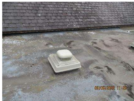
145. Extract fan external termination teaching block toilet.
