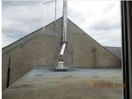
135. Boiler stainless steel chimney system.
