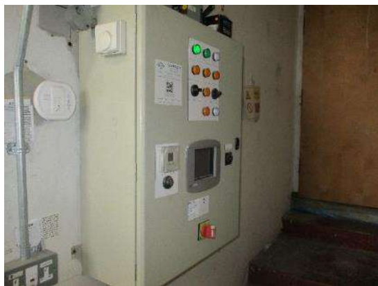
138. Heating system BEMS control panel. Teaching block.
