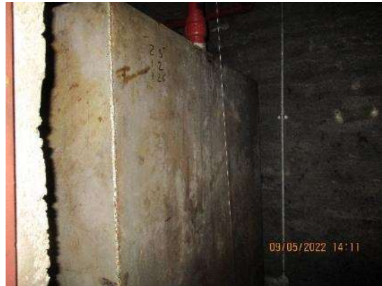
183. Oil storage tank – dining block bunded store.
