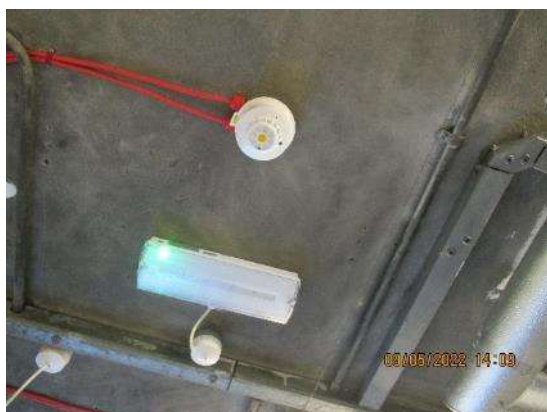
164. Fire alarm device. Detector head – teaching block.
