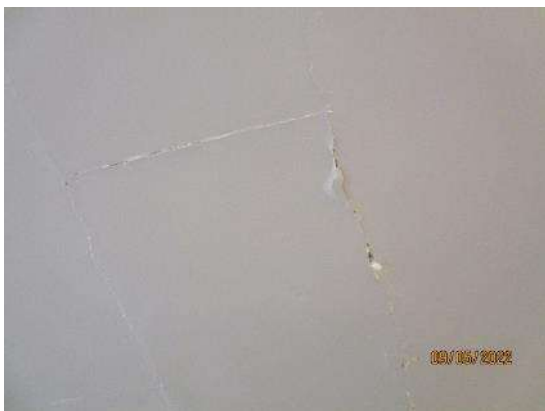
99. Plaster ceilings - cracked
