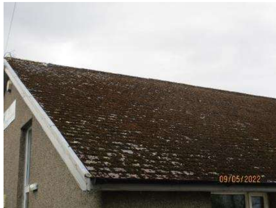
14. Asbestos tile to Teaching south
