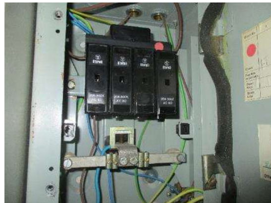
149. Electrical power – distribution board – teaching block.
