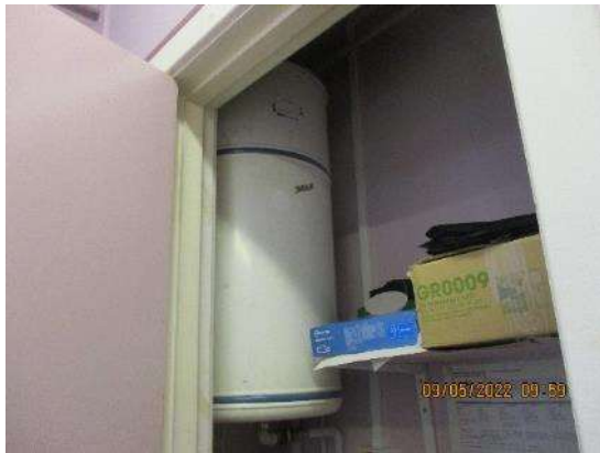
140. Hot water storage tank teaching block – electric. Girls toilets cupboard.
