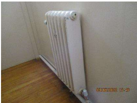
178. Radiator – dining block cloakroom.
