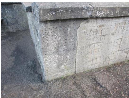
171. Perimeter wall cracking
