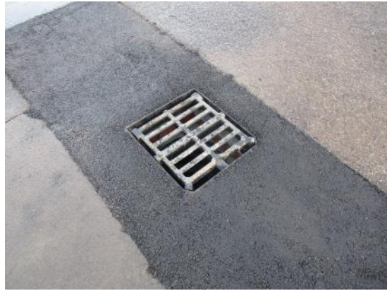
174. Surface water drainage
