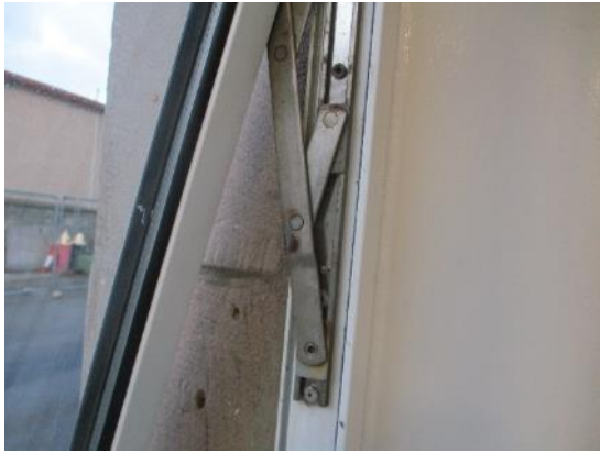
50. Window mechanisms stiff to operate
