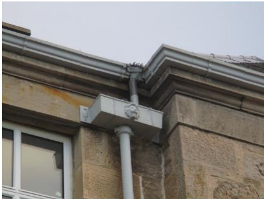
15. Previous repairs to gutter outlets
