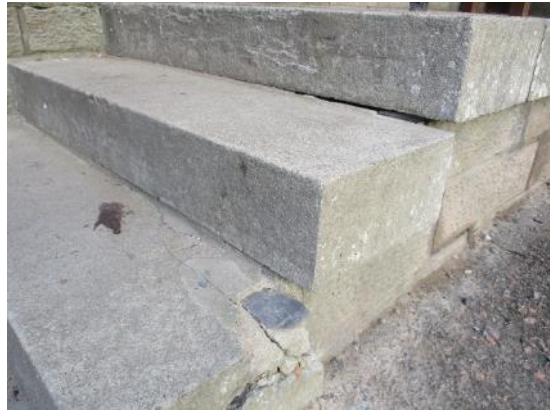
59. Damaged steps to Kitchen side door
