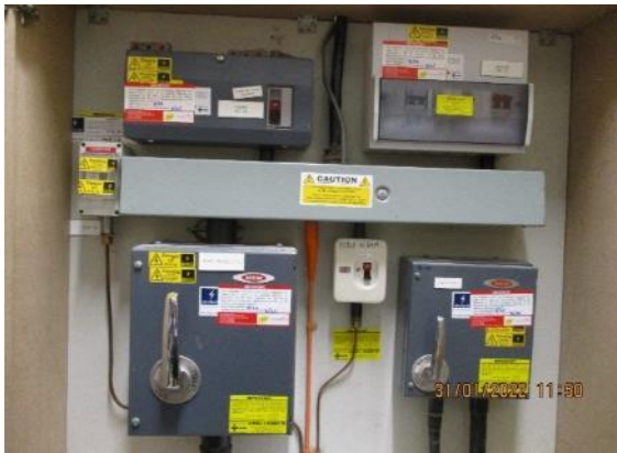
137. Electrical distribution boards and consumer unit
