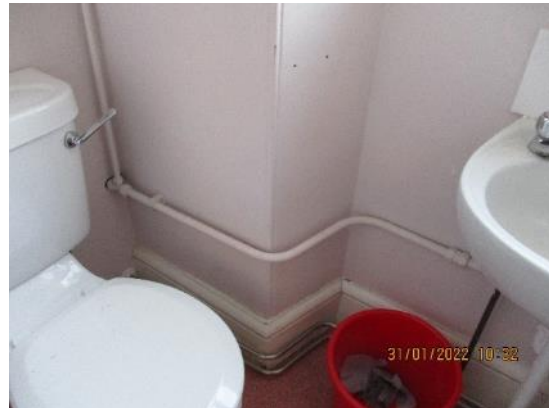
128. Cold water pipework within school building 1-36
