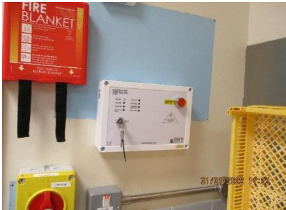
131. Automatic gas safety controls – Kitchen 1/11
