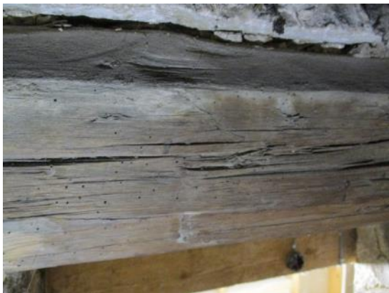
9. Woodworm in lintels
