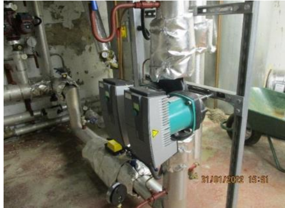
122. Plant room pumps and pipework
