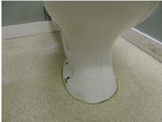
94. Cracked and chipped WC
