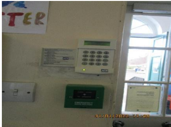
157. Intruder alarm panel – main entrance
