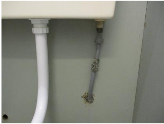
100. PVC waste pipes
