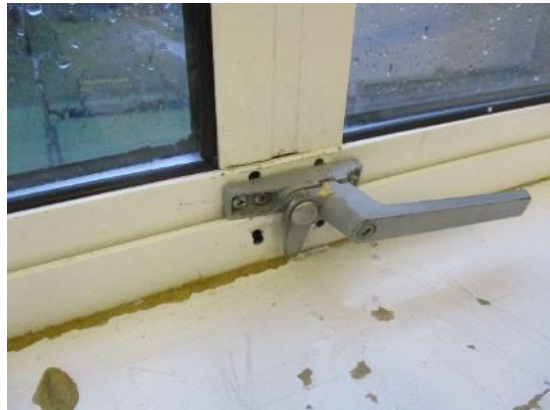
53. Lever ironmongery in very poor condition
