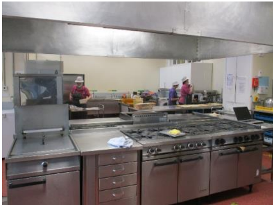
107. Stainless steel commercial kitchen
