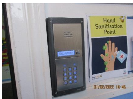
153. Door entry system
