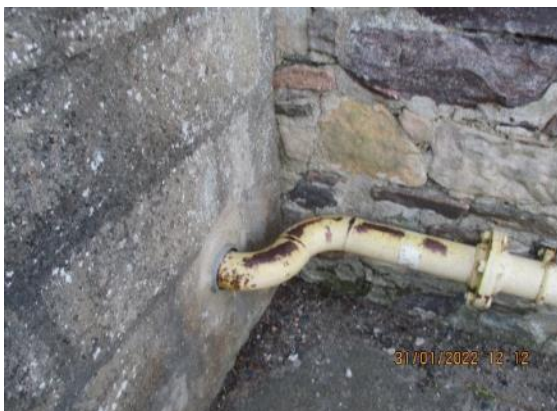
129. Gas supply to plant room – external. Main gas meter
