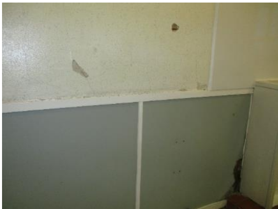
72. Isolated surface damage
