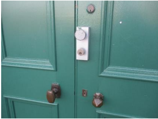
44. Door ironmongery in fair condition
