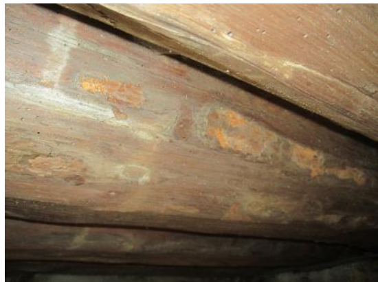
10. Woodworm in lintels
