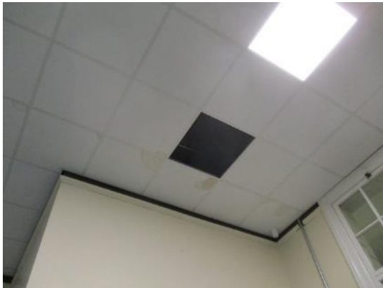
66. Water marked suspended ceiling
