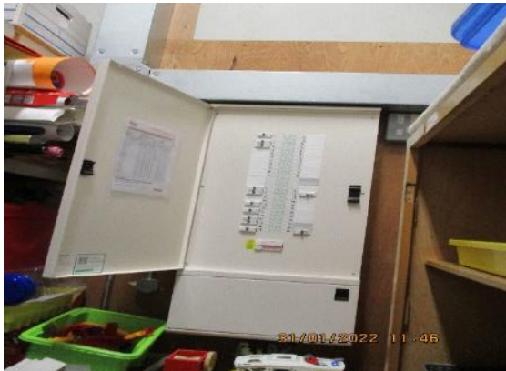
139. Electrical distribution board kitchen 1/11
