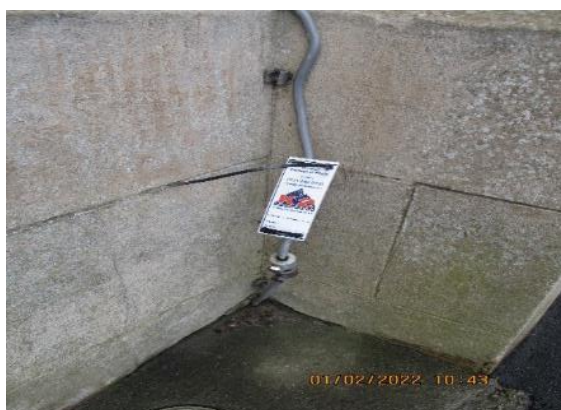
151. Lightning conductor cable ground level discharge
