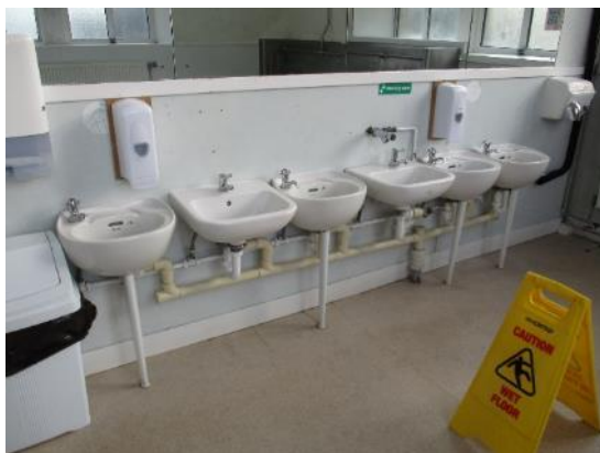
98. Typical wall hung wash hand basins
