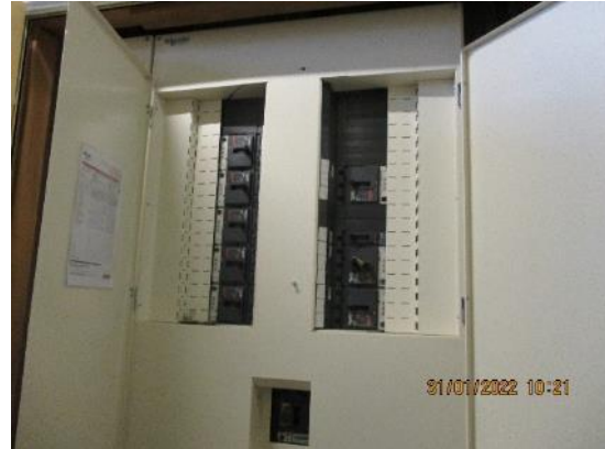
140. Electrical distribution board 2/47
