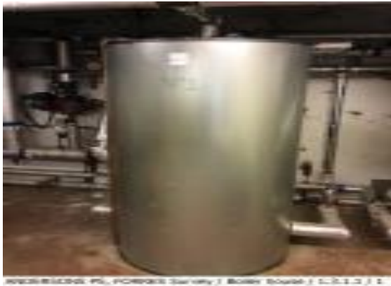
125. Hot water storage calorifier – 1 of 2 Plant room 0/29
