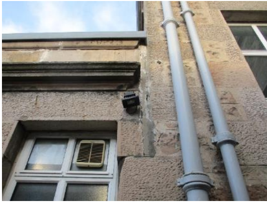
38. Isolated repointing required
