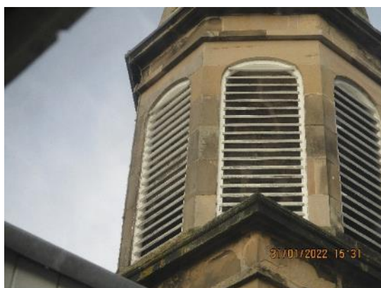
152. Lightning conductor cable clock tower
