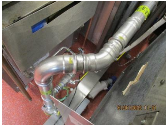
132. Gas pipework within kitchen to appliances 1/11
