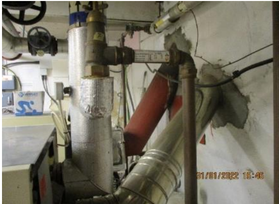
119. Boiler Flues and chimney
