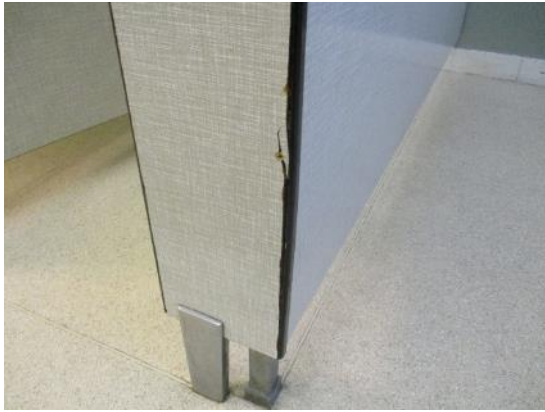
105. Damage to partitions
