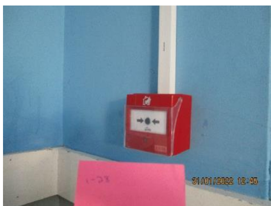
150. Fire alarm device
