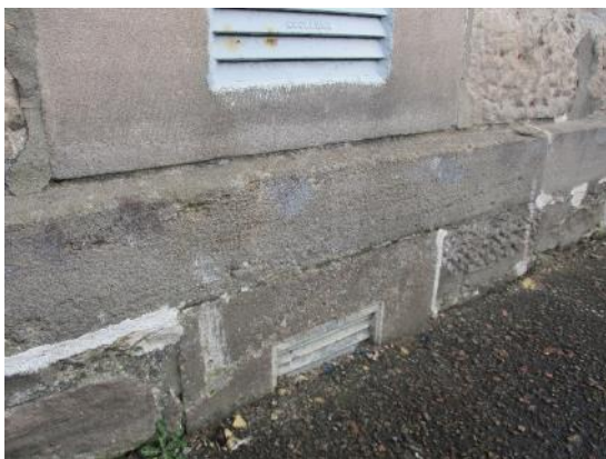
36. Under floor ventilation obstructed
