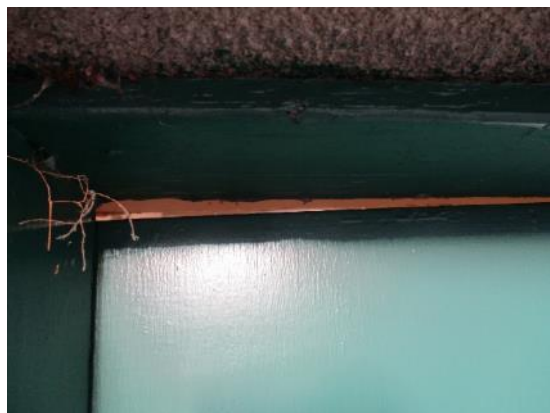
43. Door does not fit frame
