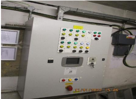
121. Plant BMS control panel and controller keypad
