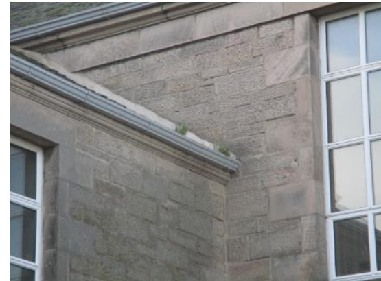
16. Vegetation in gutters
