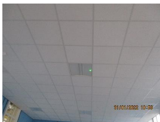
146. Emergency room lights. Non maintained Class
