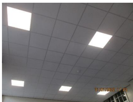
144. Classroom lighting room 1/14 / throughout.
