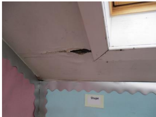
73. Plasterboard walls - Water damage
