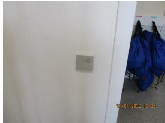
156. Disabled alarm system call point – access toilet
