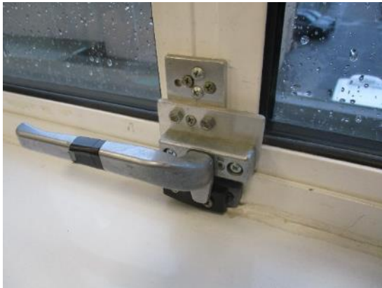
52. Lever ironmongery in very poor condition
