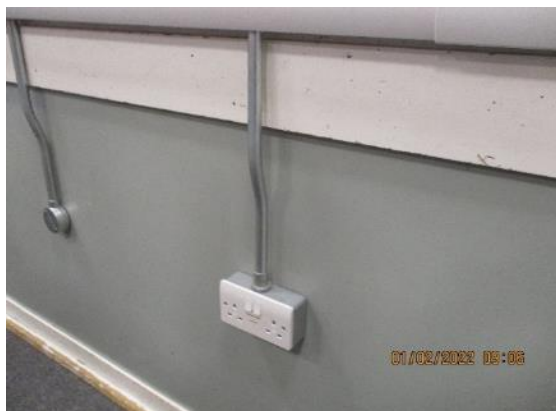
141. Wiring accessories and conduit and trunking-classroom
