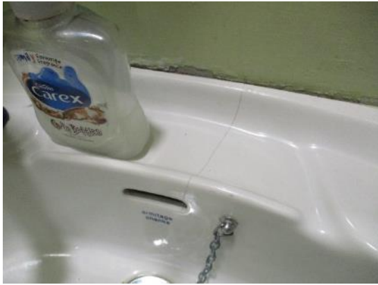
99. Cracked wash hand basins
