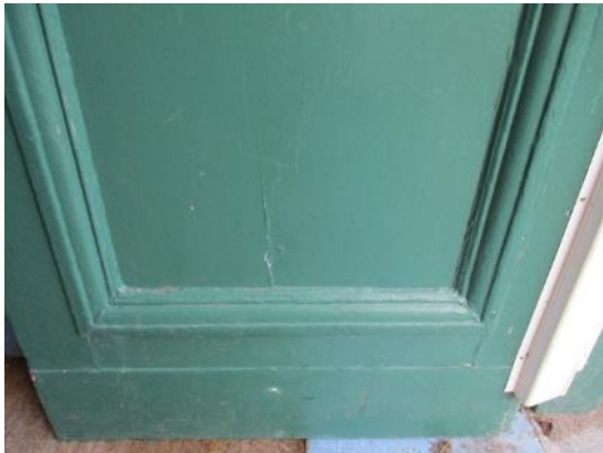
40. Isolated repairs required
