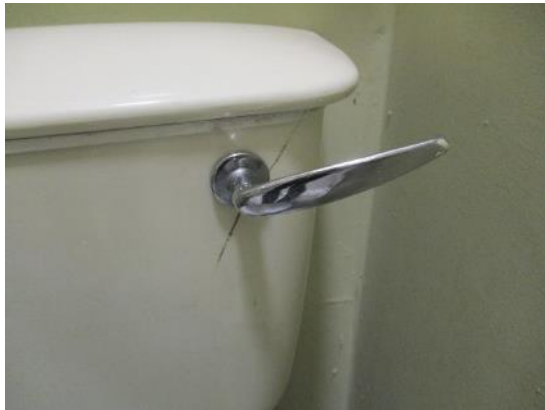
96. Cracked vitreous china cisterns
