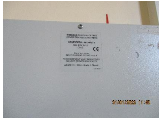
158. Intruder alarm panel main entrance
