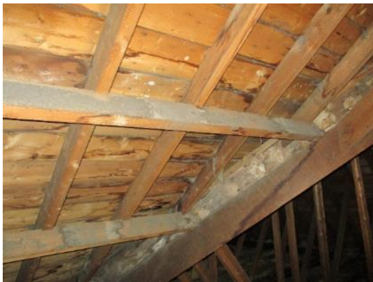
6. Water marked timbers
