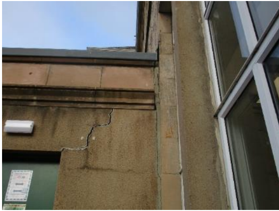
32. Movement and cracking of external walls
