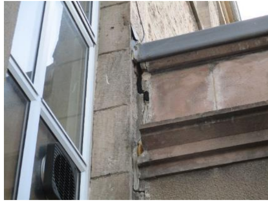
33. Gap between the extension and the main building
