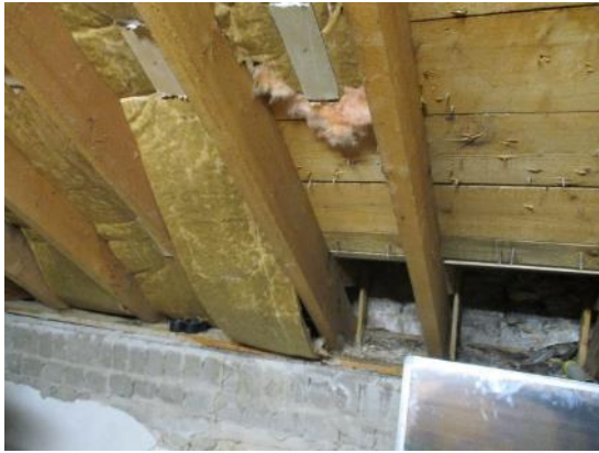
13. Damaged/missing insulation to north roof
