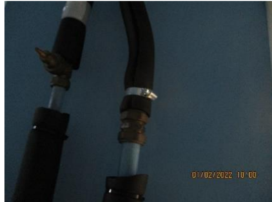
126. Hot water pipework within school building
