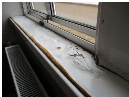
81. Water damaged MDF window linings
