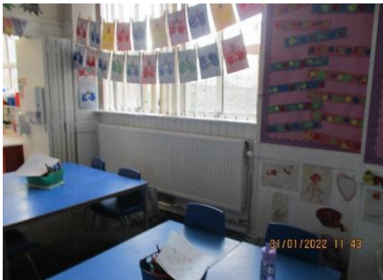
123. Typical heating system radiator
