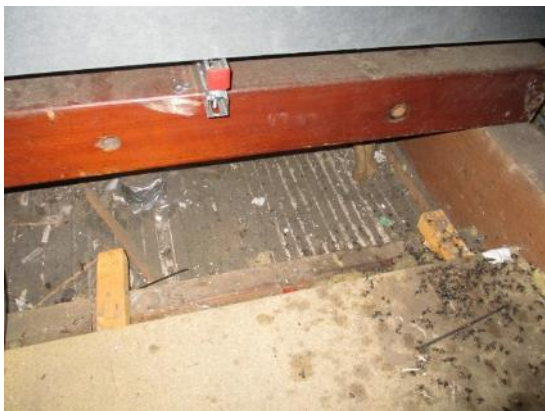
11. Disturbed/missing mineral insulation
