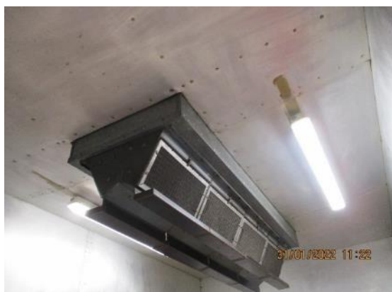
135. Specialist extract mechanical ventilation kitchen 1/11
