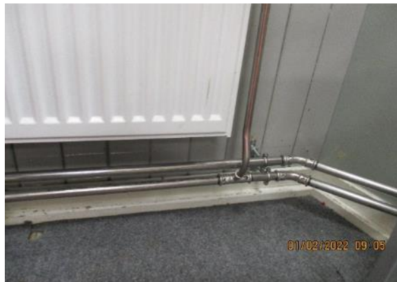
124. Heating system pipework
