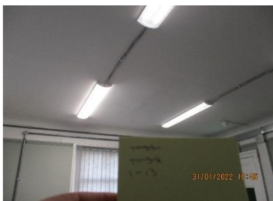
143. Office lighting HT – Room 1/13
