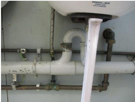
101. Copper waste pipes
