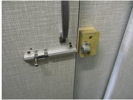
106. Failed and repaired ironmongery
