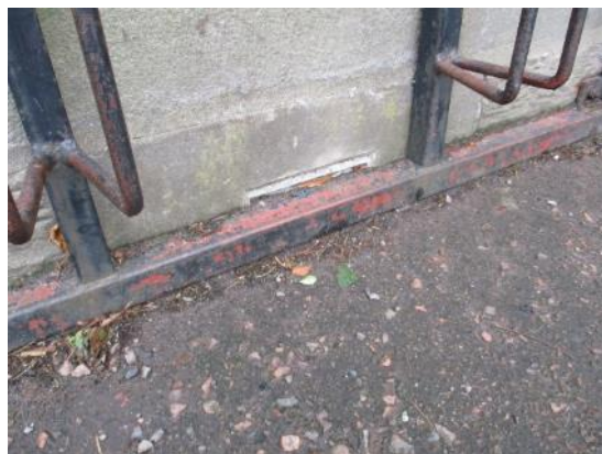
37. Under floor ventilation obstructed
