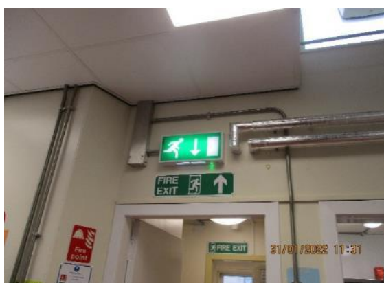
145. Emergency exit maintained lighting kitchen 1/11
