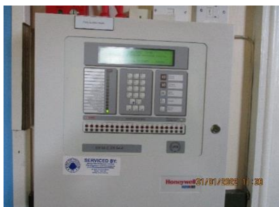
149. Fire alarm panel
