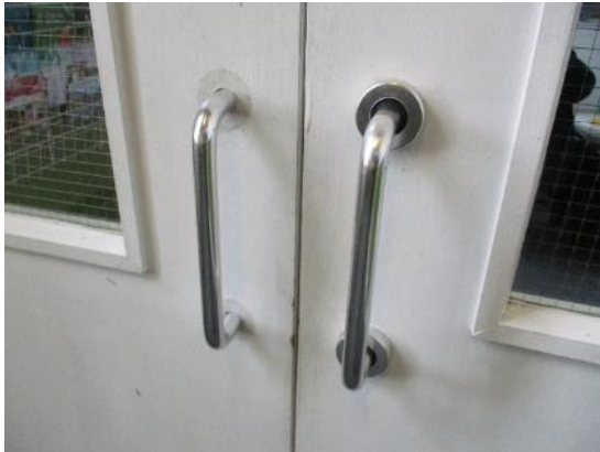
88. Isolated missing ironmongery
