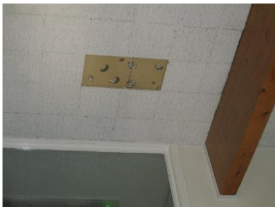
69. Ceiling tiles failing
