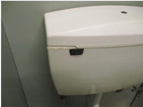
95. Damaged plastic cisterns
