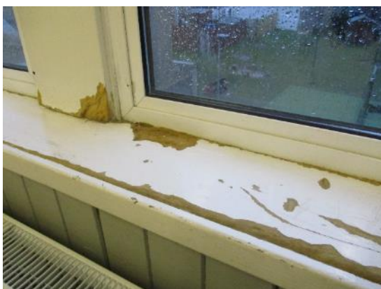
80. Water damaged MDF window linings
