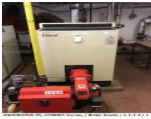
120. Cast iron sectional gas boiler 1 of 2
