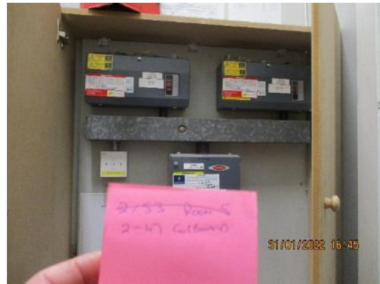
138. Electrical distribution boards
