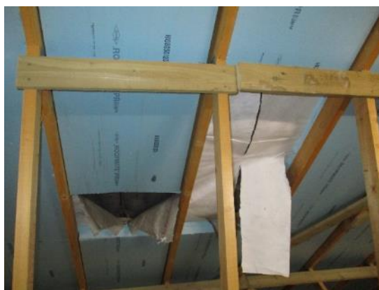
20. Damaged insulation below tiles
