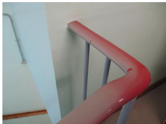
66. Faded PVC handrail covers
