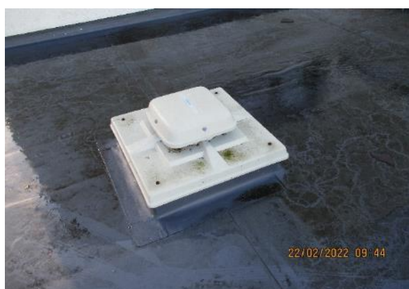
157. Roof – extract fan termination.
