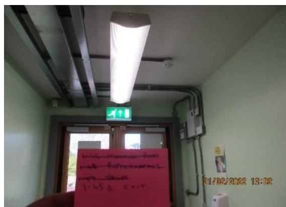
138. Emergency lighting – maintained fire exit
