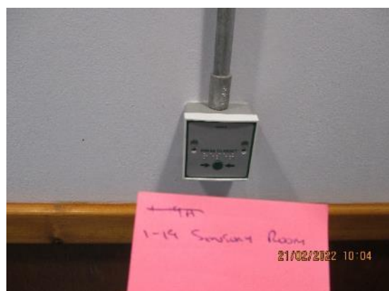
148. Communication systems. Accessible toilet alarm system.
