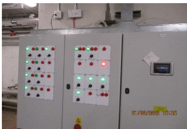
125. BMS control panel – Plant room
