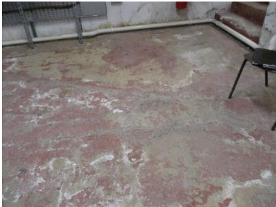
57. Painted concrete floor – Boiler House
