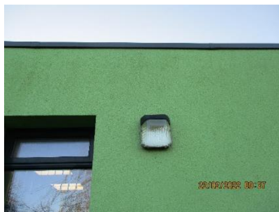
140. External building lighting
