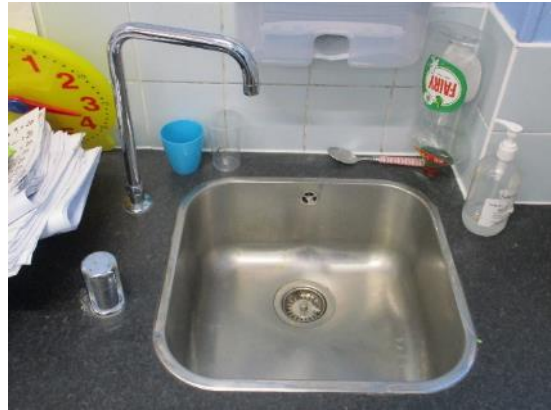
104. Classroom stainless steel sink
