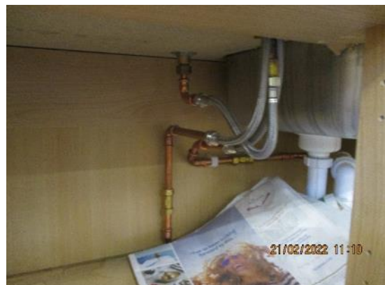
116. Hot water copper pipework classroom sink
