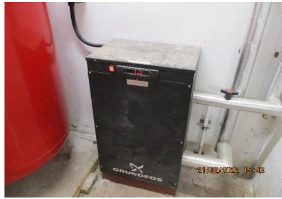
112. Pressurisation Unit – Heating system
