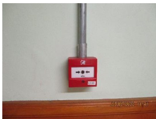
142. Fire alarm device – call point.
