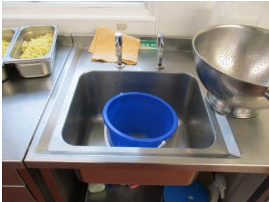
103. Commercial kitchen sink
