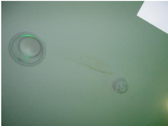
69. Water mark in Soft Play Room
