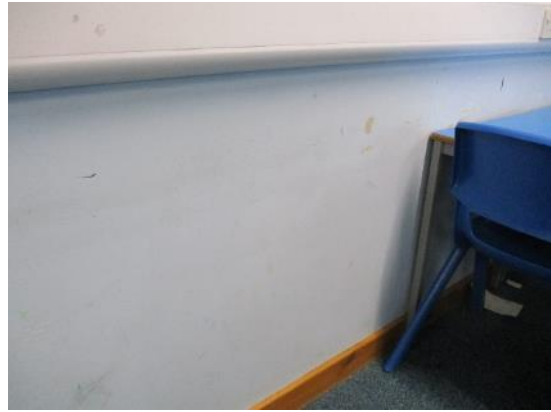
74. Damaged plastered walls
