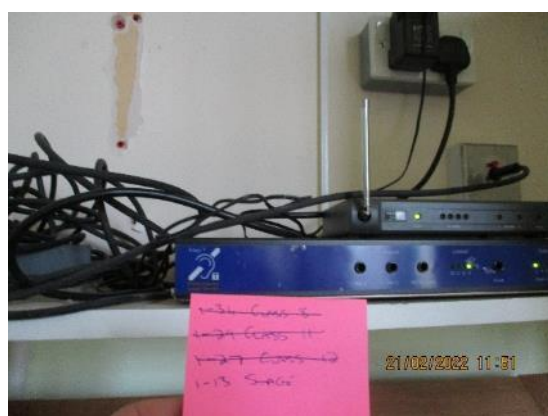
145. Communication systems – Hearing induction loop system unit.
