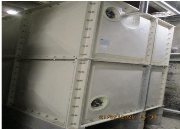
117. Cold water tank – plant room
