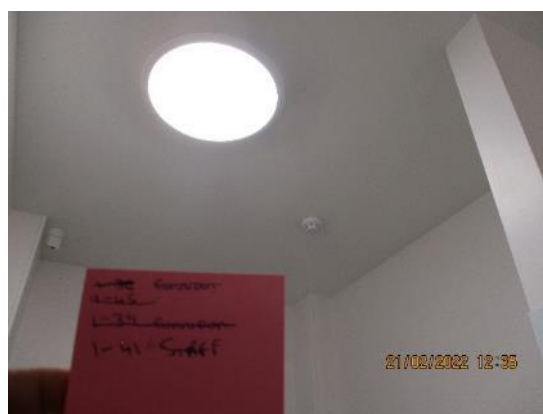
136. Lighting – toilets and stores
