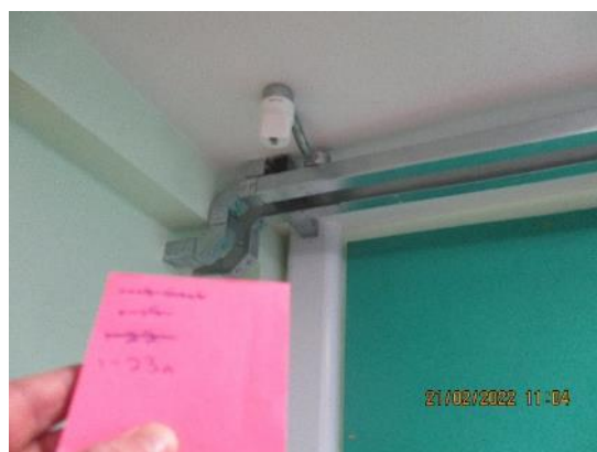
132. Lighting control – PIR motion sensor.
