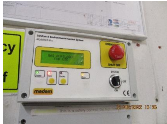
120. Gas safety auto shut down control panel
