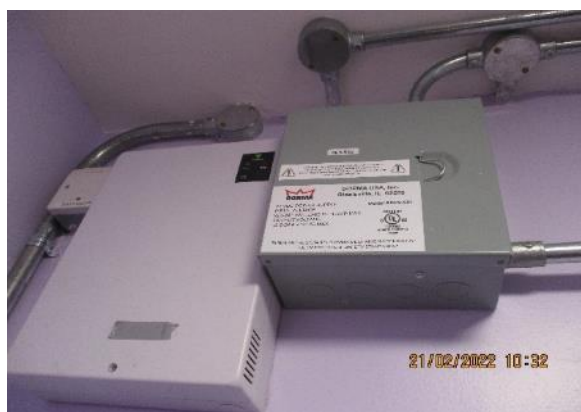
143. Fire door internal auto close control system.
