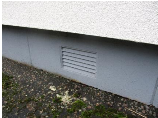
32. Under floor ventilation
