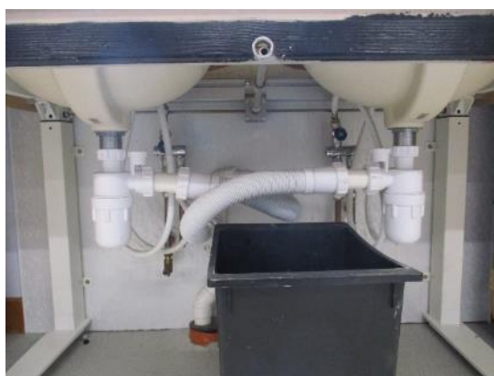
94. PVC waste pipes
