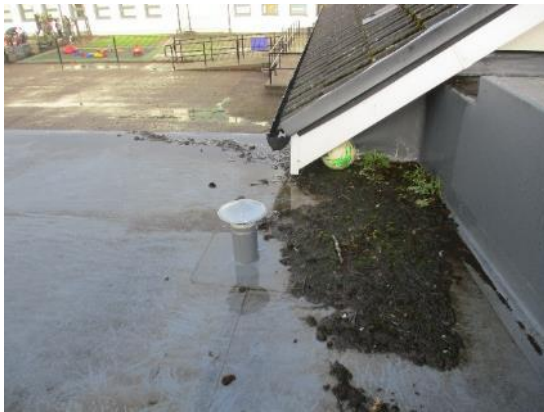
13. Debris and vegetation
