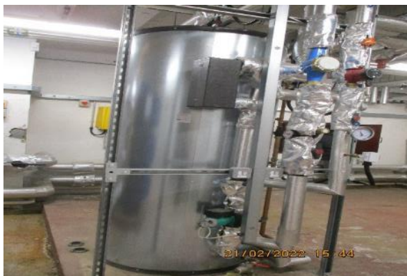
115. Hot water storage calorifier
