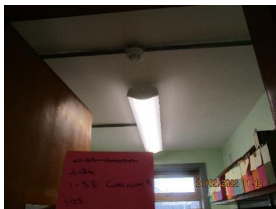
144. Fire alarm detector head.
