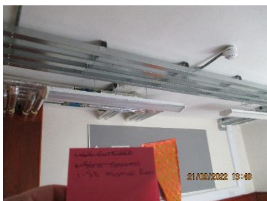
129. General wiring within metal protective trunking.
