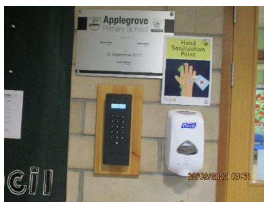
146. Communication systems. Entrance door audio intercom system.
