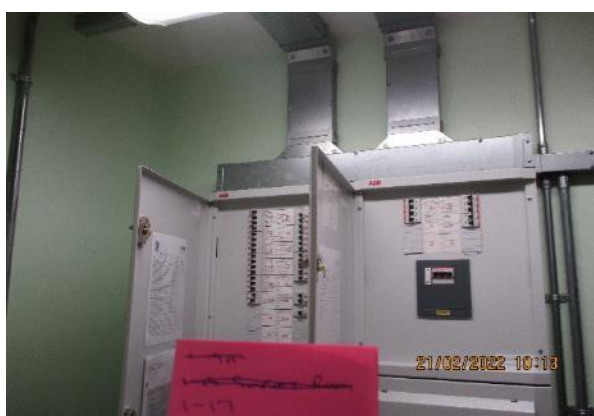
127. Distribution boards – lighting and power
