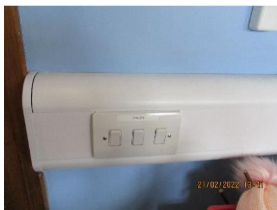
130. General wiring within protective plastic trunking.
