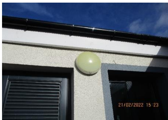
139. External building lighting.
