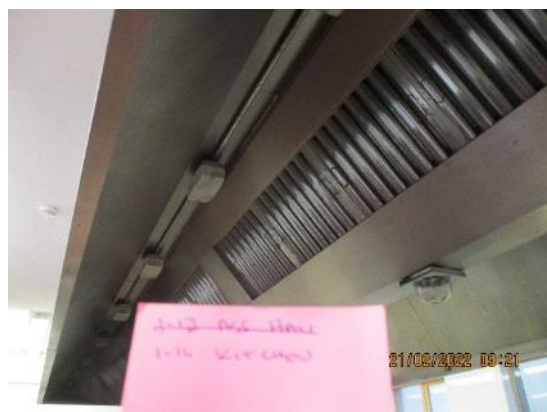
124. Specialist ventilation. Kitchen appliance canopy
