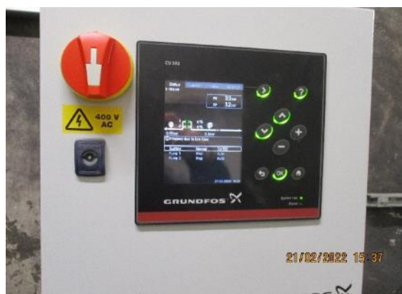
126. Control panel – cold water booster pump
