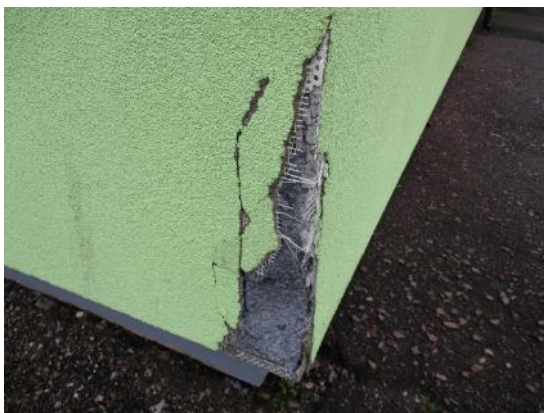
35. Damage to external insulation
