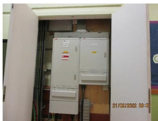
128. Distribution boards – lighting and power
