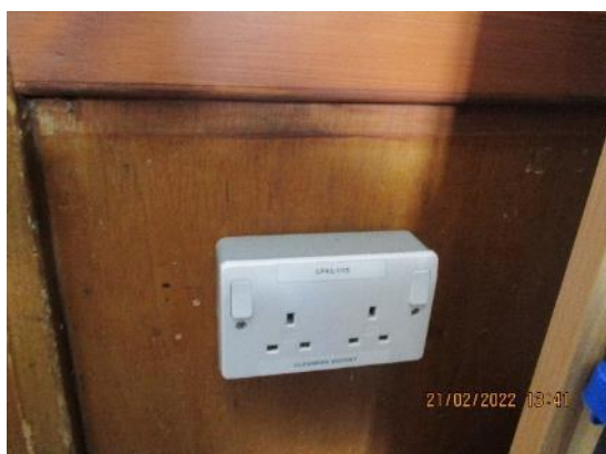
131. Wiring accessories. Surface socket metal back box.
