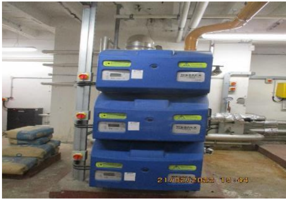
111. Gas boilers – Modular (3 of)
