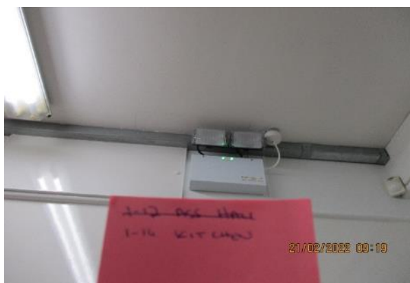
137. Emergency lighting kitchen.
