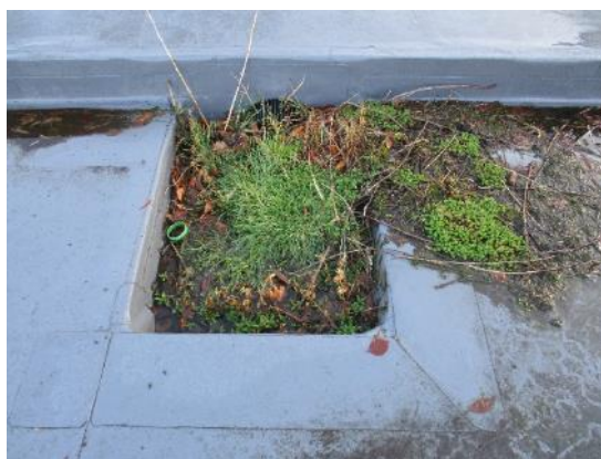
24. Blocked flat roof outlets
