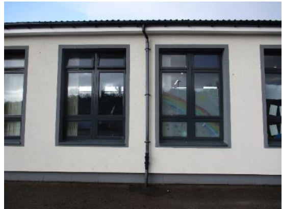
28. UPVC rainwater downpipes
