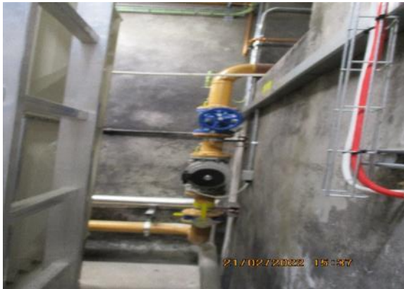
119. Gas supply pipework and electric solenoid control.
