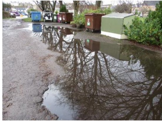
160. Surface damage and flooding
