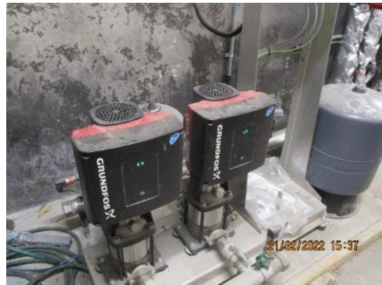
118. Cold water booster pump set.
