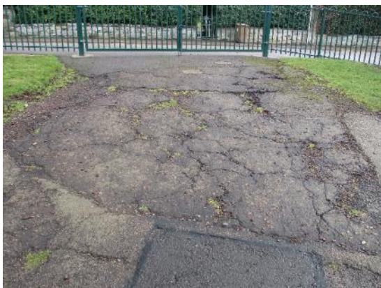
163. Damaged tarmacadam at gates
