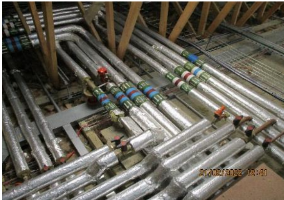
113. Heating pipework and insulation – attic space
