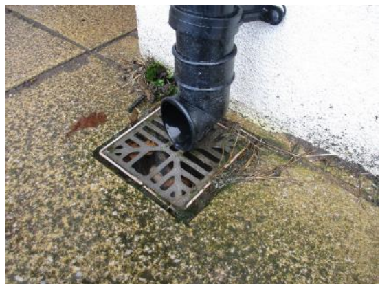
30. Surface water gullies
