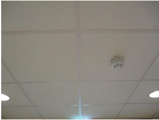
67. Suspended ceiling tiles
