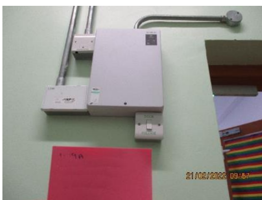
152. Security – door access control system. Paxton.
