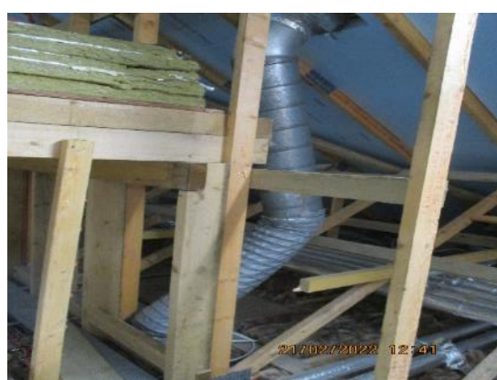
158. Attic space extract fan ductwork.
