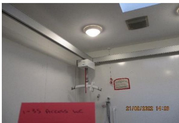
155. Lifts and hoists. 200kg Person hoist.
