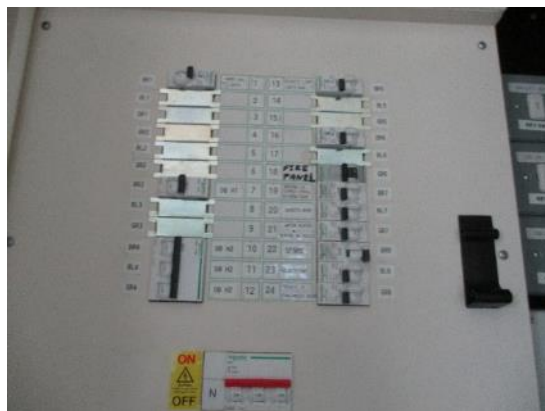
61. Main school distribution board.
