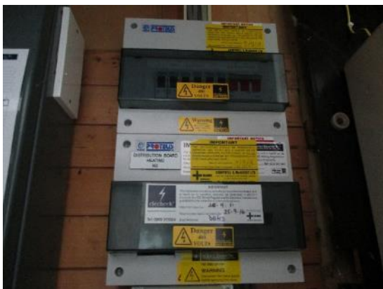
60. Kitchen block distribution boards.
