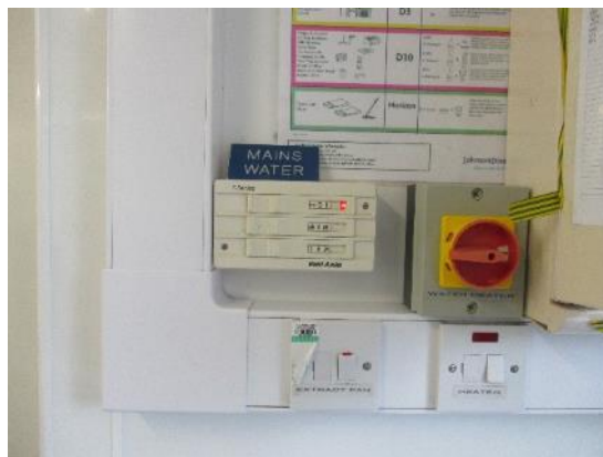
42. Specialist ventilation controls - Kitchen
