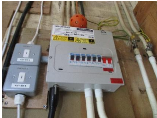
59. Horsa Hut distribution board.
