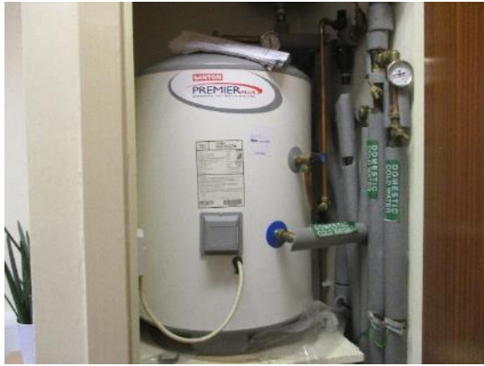
37. Hot water cylinder main school
