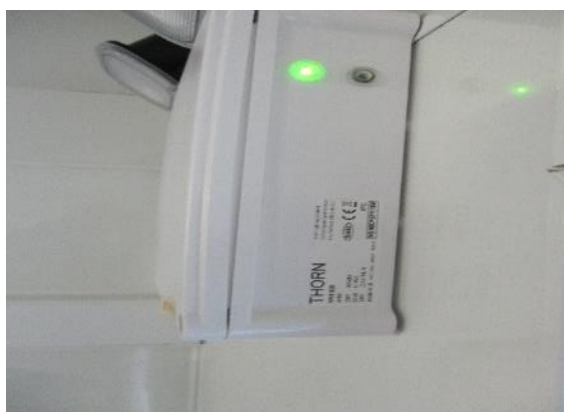
48. Emergency lights kitchen.
