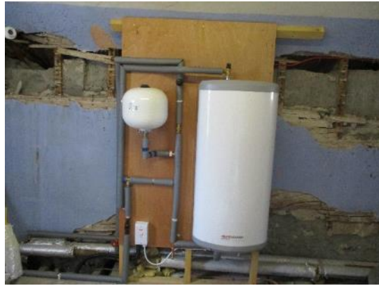
38. Multipoint hot water storage heater - kitchen
