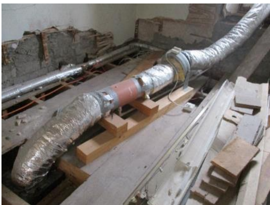
41. Specialist extract ventilation – Kitchen
