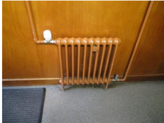
32. Cast iron radiator main school
