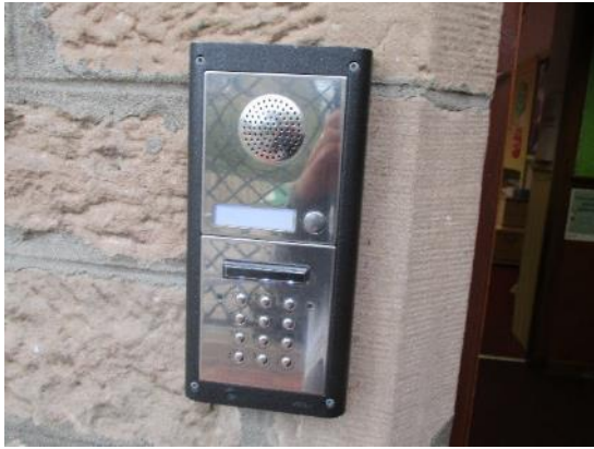
56. Main entrance door entry system call.
