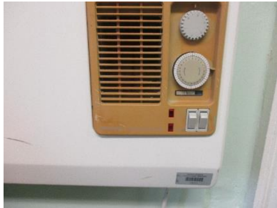
34. Kitchen block electric convector heater
