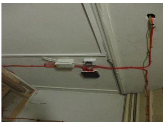
46. Fire alarm system wiring attic main school.
