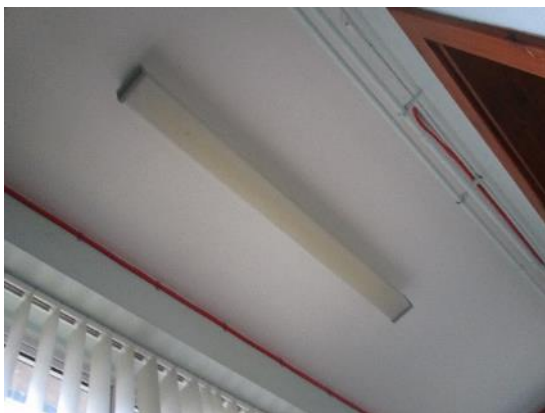
54. Main school reception batten light.
