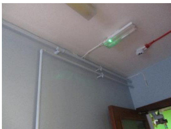
47. Emergency lights main school.
