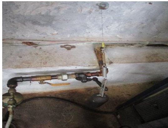
40. Oil supply pipework to boiler – Plant room
