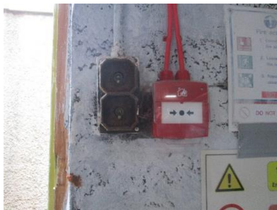
55. Main school plant room light switches.
