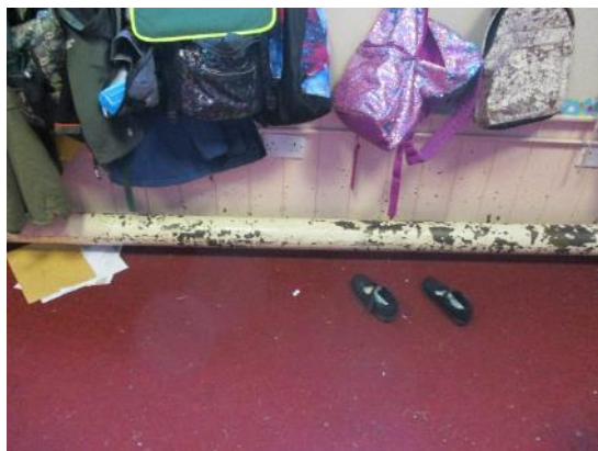
35. Heating pipe main school
