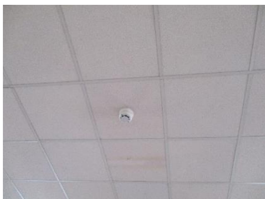
45. Fire alarm system detector head.
