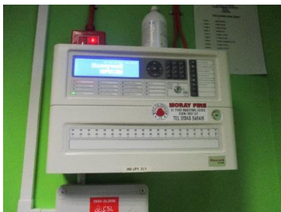
43. Fire alarm panel. Main school
