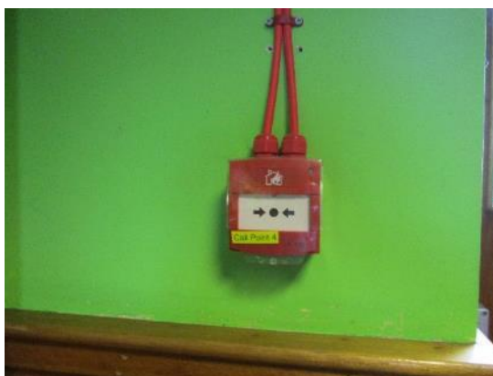
44. Fire alarm system device – call point main school.
