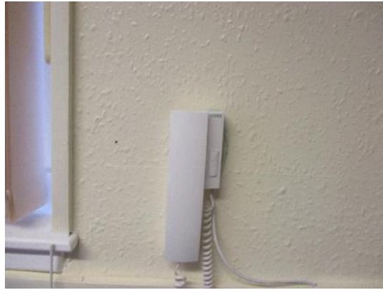
57. Main entrance door entry receiver.
