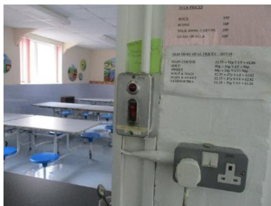
74. Kitchen sockets and switches
