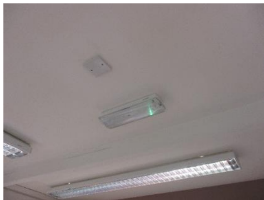
30. Main school lighting and emergency lights
