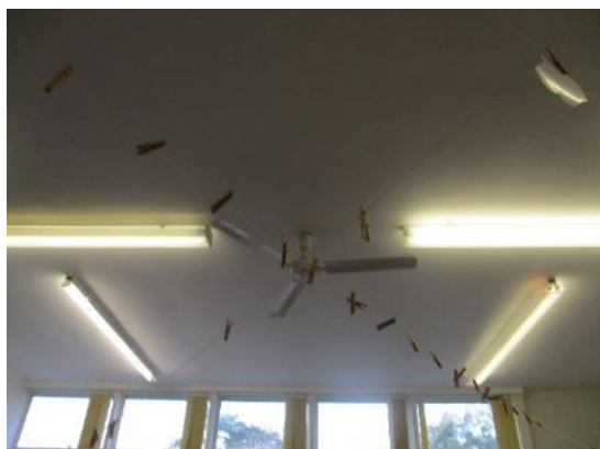
33. Main school class lighting
