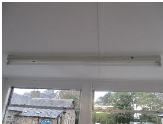
36. Main school Portacabin lighting
