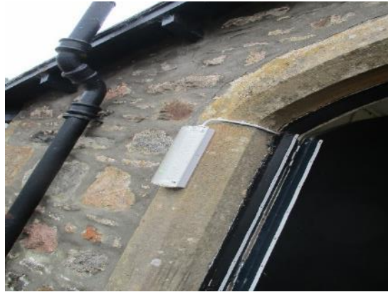
58. External emergency light.
