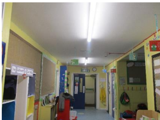
34. Main school corridor lighting
