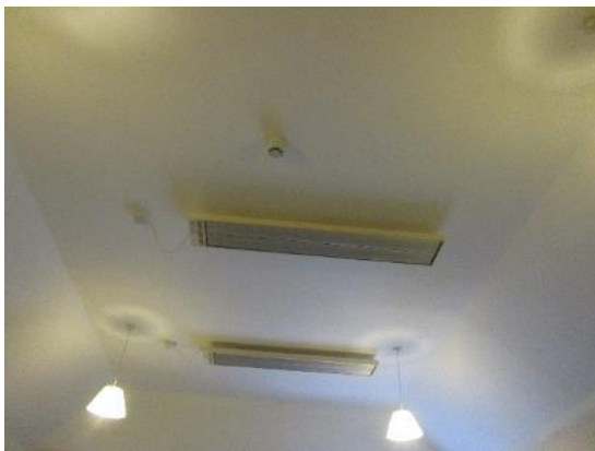
59. Hall store radiant panel heaters and lights.
