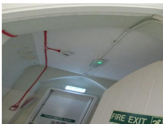
32. Fire alarm system wiring and devices.
