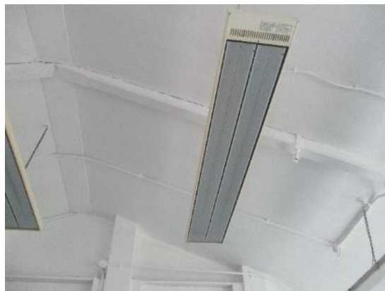
60. Hall radiant panel heaters
