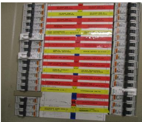
29. Main school distribution board
