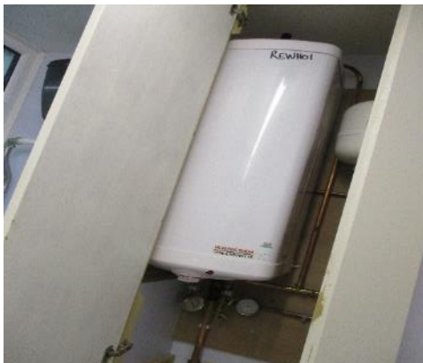
27. Boys toilet multipoint water heater
