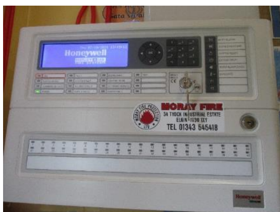
31. Main school fire alarm panel
