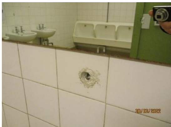
68. Damaged wall tiles
