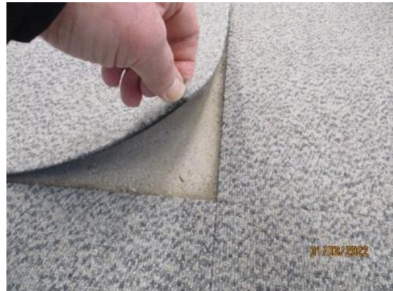
57. Carpet tiles loose and lifting
