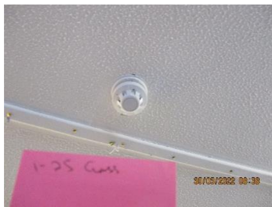
126. Fire/smoke detector head – classroom 1/25
