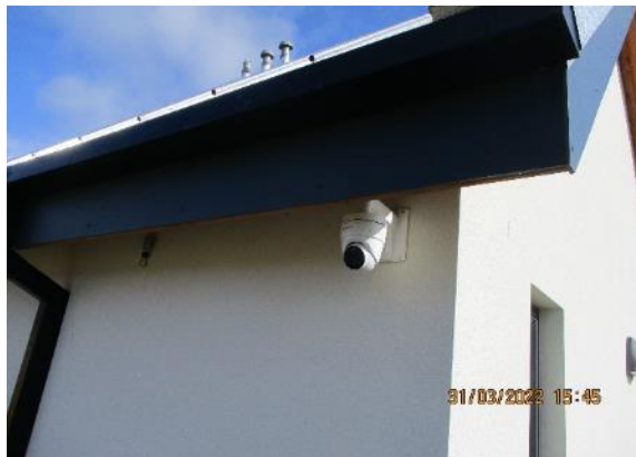
157. CCTV Camera external
