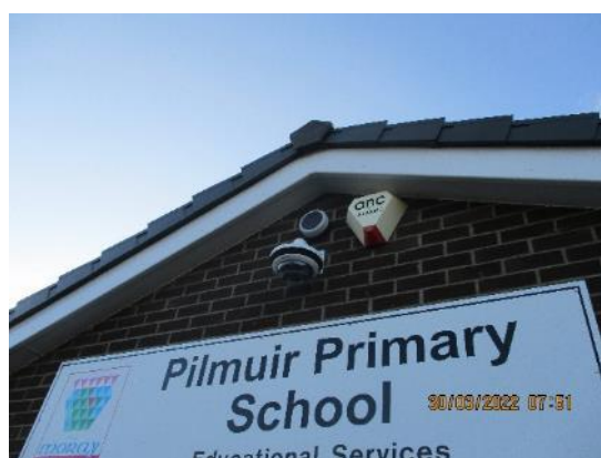
130. CCTV fixed camera main entrance.
