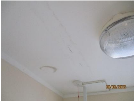
60. Failed taped joints
