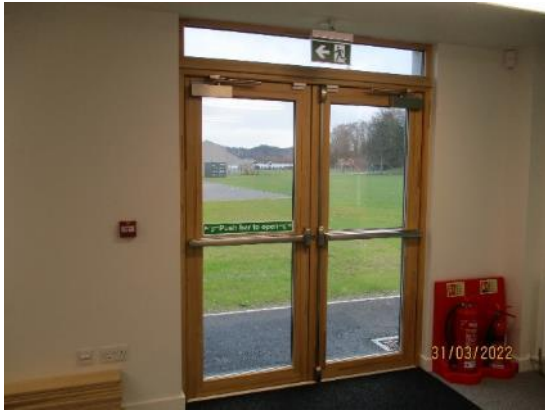
31. Fire exit ironmongery
