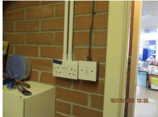
120. Switches and sockets typical
