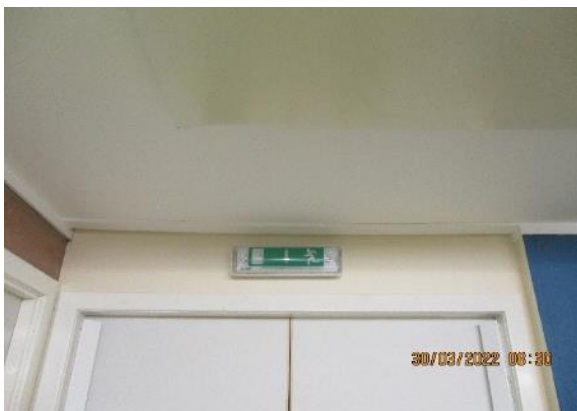
123. Emergency exit light.
