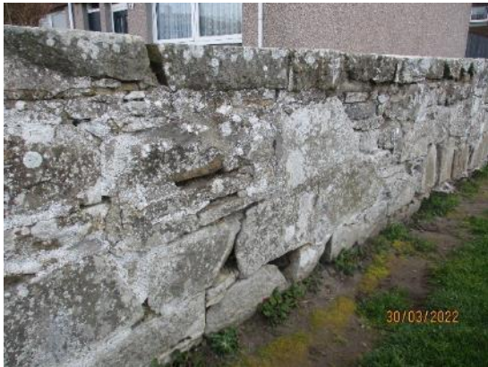
181. Stone wall repairs and repointing required
