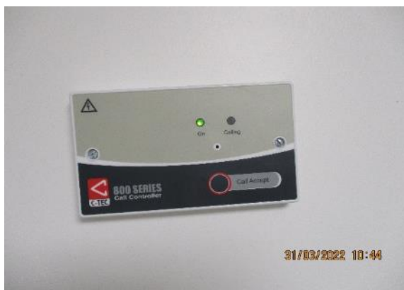
159. Disabled toilet alarm indicator panel
