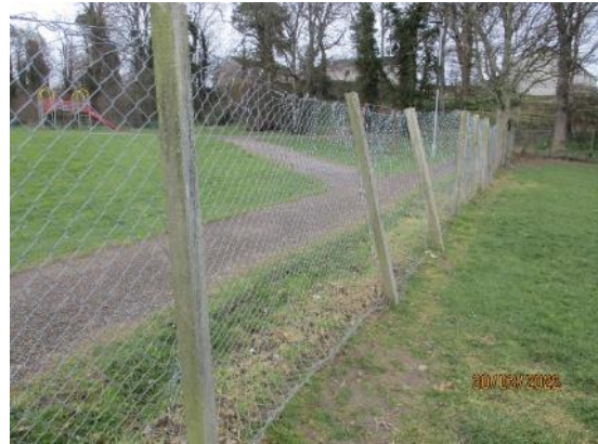
174. Leaning concrete posts to playing field
