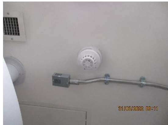
152. Fire alarm – detector head.
