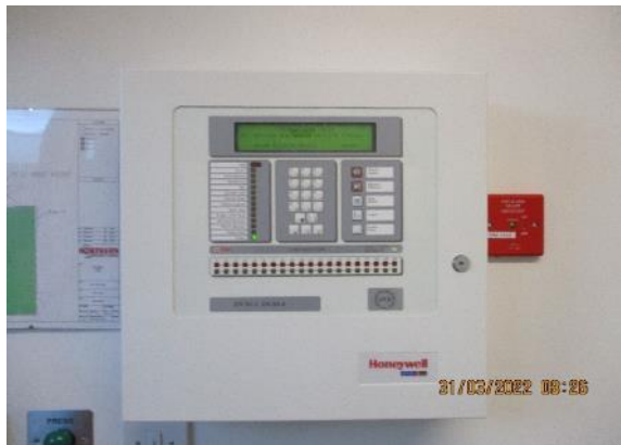
151. Fire alarm panel
