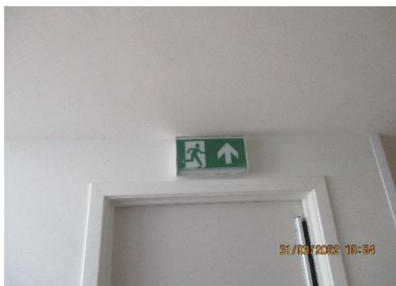
153. Emergency exit sign light.
