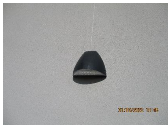
160. External lighting typical
