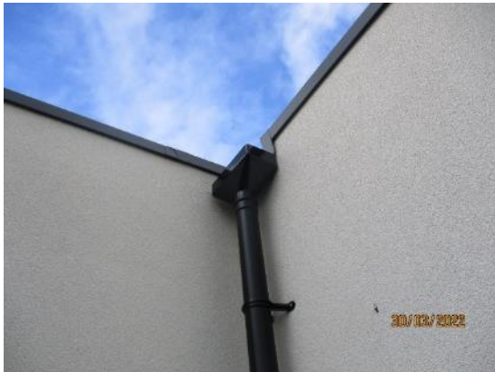
15. Annexe hopper heads & downpipes
