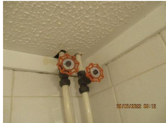
110. Hot water pipework typical
