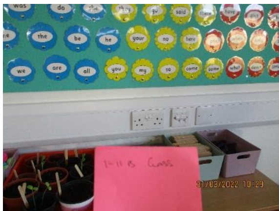
147. Sockets and switches
