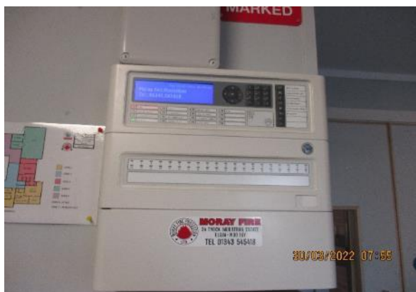
125. Fire alarm panel – entrance lobby
