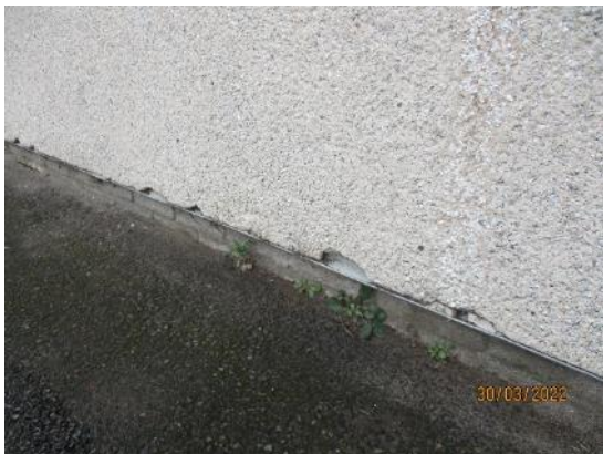
21. Spalling at bellcast bead
