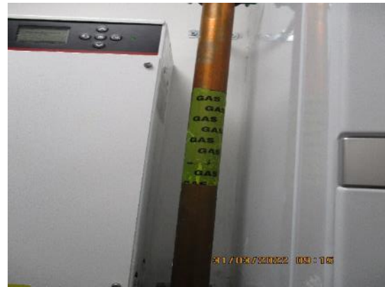
144. Gas pipework plant room.
