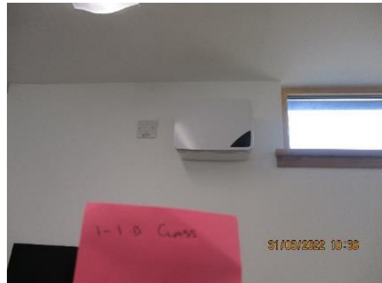
146. Extract fan - classroom
