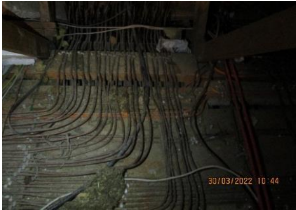
119. General wiring – attic space
