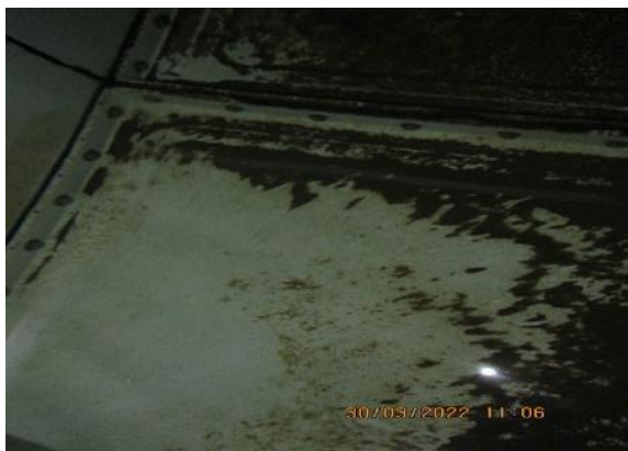
111. Cold water tank internal – attic space
