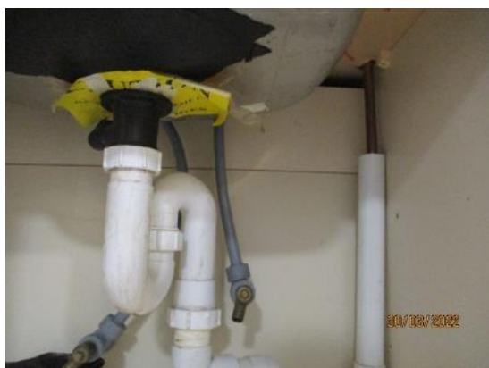
84. PVC waste pipes
