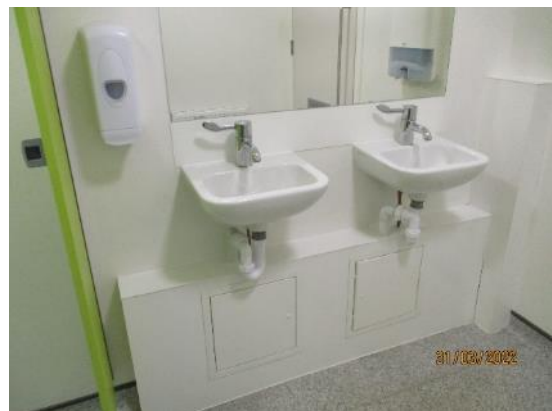
83. Typical Annexe wall hung basins
