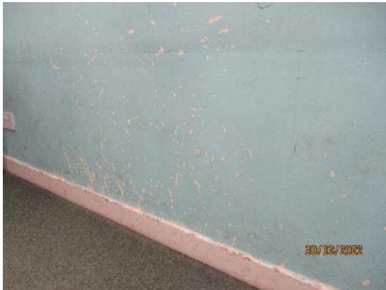
98. Chipped and peeling internal decoration
