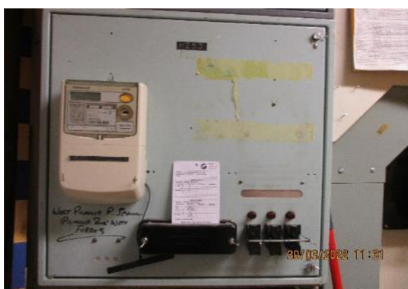
117. Incoming power supply and meter board.
