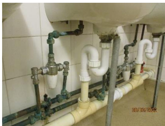
85. PVC waste pipes faded and discoloured
