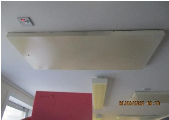
107. Electric ceiling radiant heater panels circulation.
