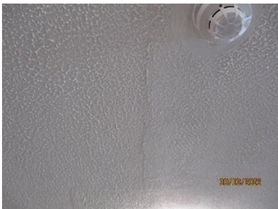
58. Textured ceilings – cracking at taped joints
