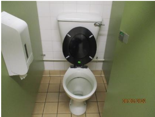
80. Typical Primary WC
