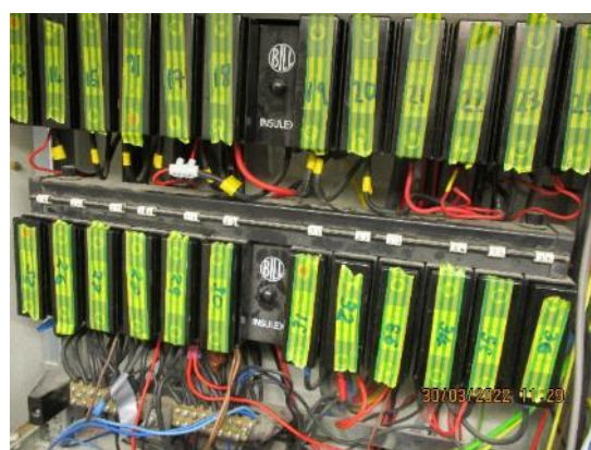
118. Distribution board – switchgear room
