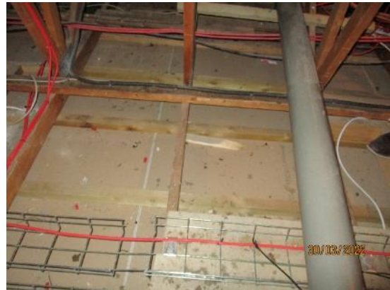
10. Lack of insulation
