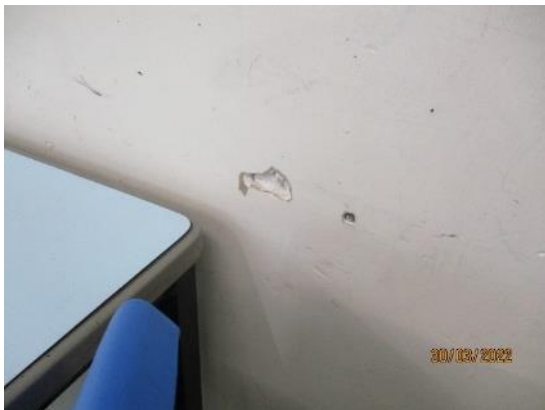
62. Isolated areas of surface damage
