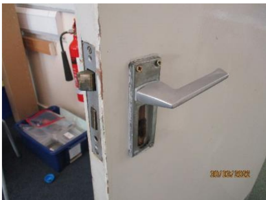
76. Ironmongery – repairs required
