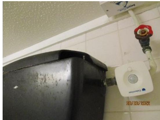
79. Damage to high level cisterns
