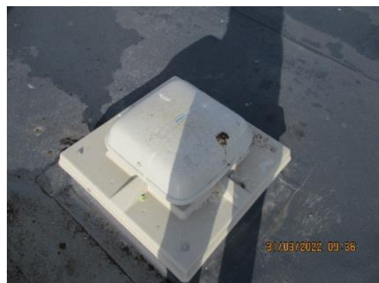
166. Extract fan terminal – roof.
