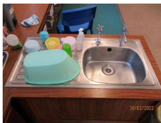
95. Stainless steel sinks with pillar taps
