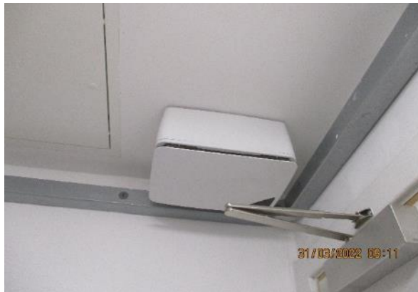
145. Extract fan – plant room
