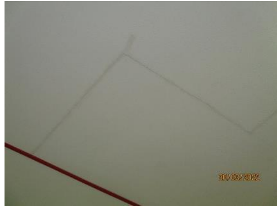
61. Plasterboard open joints
