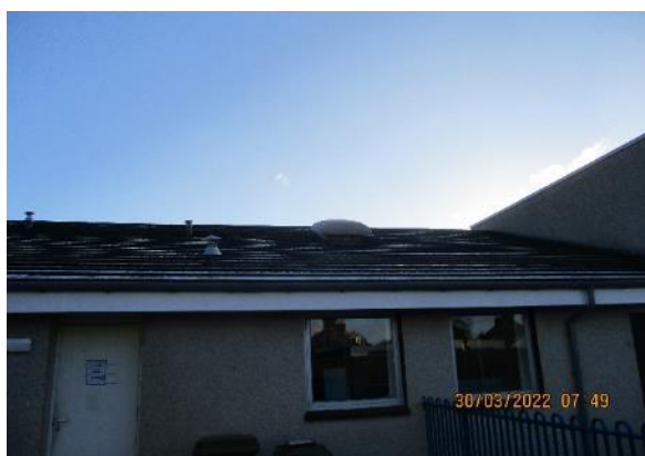
115. Kitchen extract specialist fan terminal.
