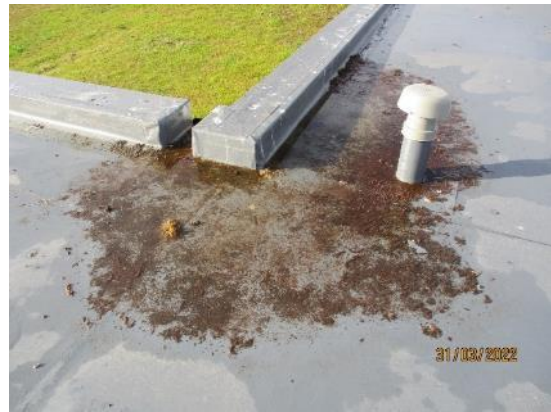
8. Inadequate falls to outlets
