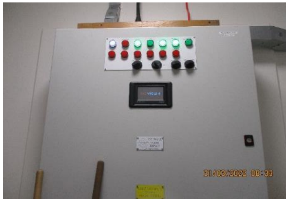
139. Building management system control panel.
