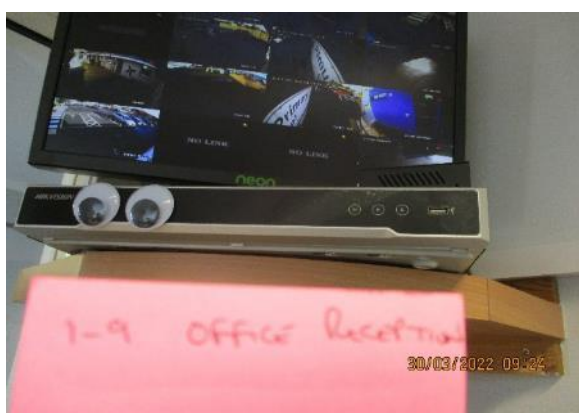
129. CCTV monitor and recorder. Reception office.
