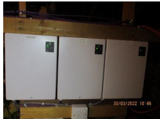
134. Paxton security door control units. Attic space.
