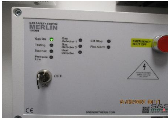
143. Gas safety system control panel plant room.
