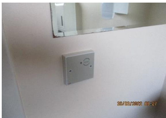
135. Disabled toilet alarm system push pad – access WC
