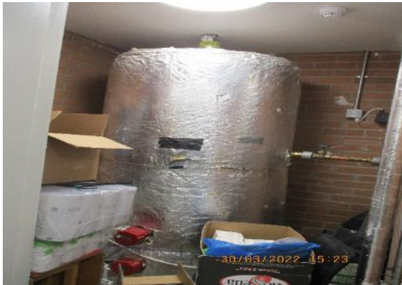
109. Hot water storage calorifier
