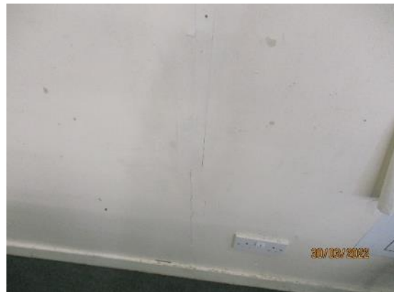
63. Plasterboard taped joints failing
