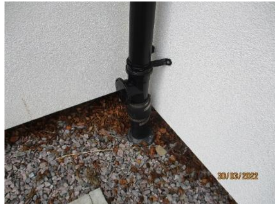
16. Discharging below ground
