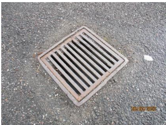
183. Road gully car park drainage
