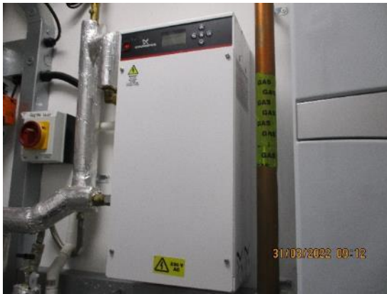
137. Heating system press unit and boiler. Plant room.
