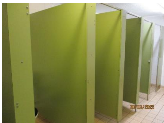
88. Primary cubicle partitions
