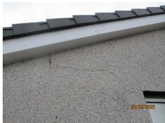
18. Cracks in masonry
