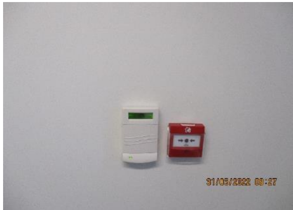
155. Intruder alarm control panel main entrance
