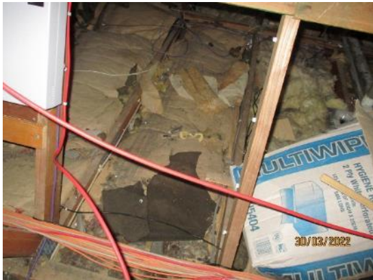
9. School loft insulation – thin & patchy
