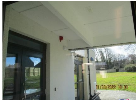
158. CCTV external camera rear exit door
