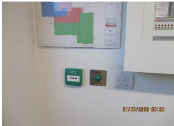
163. Security door release buttons and emergency release
