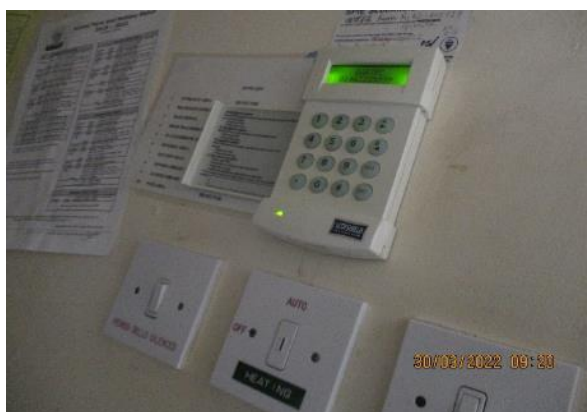
127. Intruder alarm panel. Reception store.
