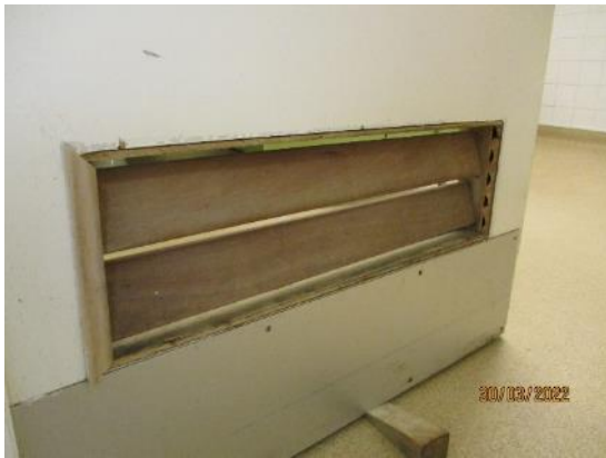
72. Isolated areas of damage to timber doors
