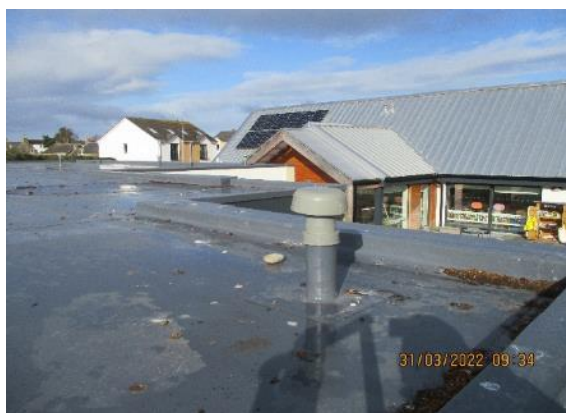
165. Extract fan terminations roof view
