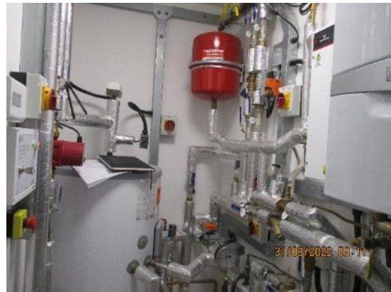
138. Heating system pipework and controls.
