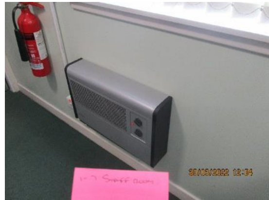
108. Electric convector heater – staff room.
