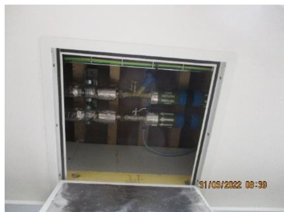
142. Hot and cold water domestic pipework
