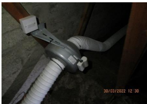
113. Extract fan – girls toilets. In line in attic space
