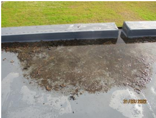
7. Part blocked rainwater outlets
