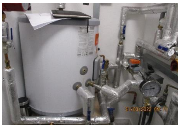
141. Hot water storage cylinder and pipework.
