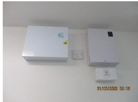
164. Security door control system panel
