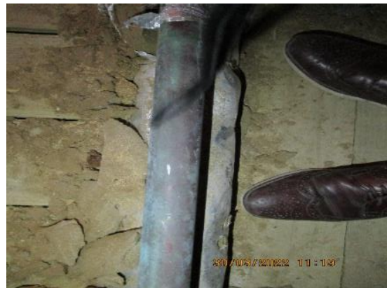
112. Cold water pipework attic space
