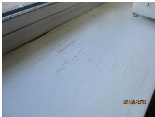
69. Timber window sills, cracking and peeling
