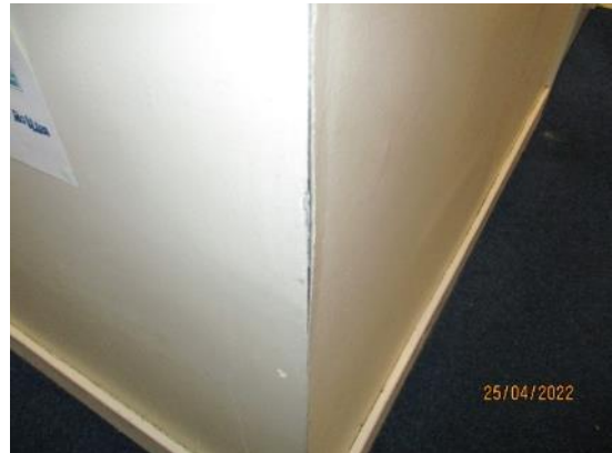
104. Damaged plasterboard walls
