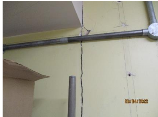
98. Dining Hall cracked walls
