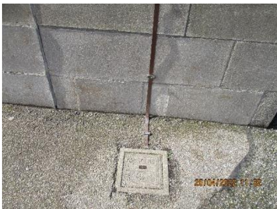
175. Lightning conductor cable and earth rod.
