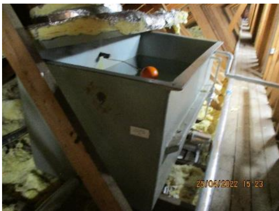
151. Cold water storage tank – attic.
