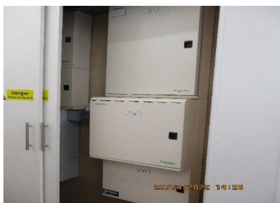
205. Distribution boards – power. 1/40 kitchen cupboard.
