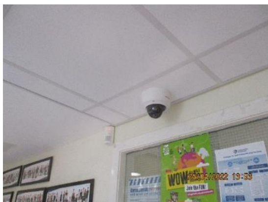
183. CCTV system fixed camera. Internal at reception.
