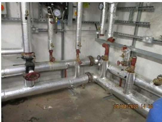
145. Pipework – heating system. 0/1 Boilerhouse.
