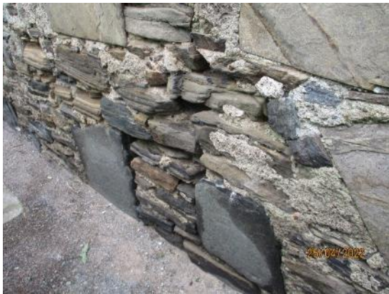
237. Repointing of stone walls required
