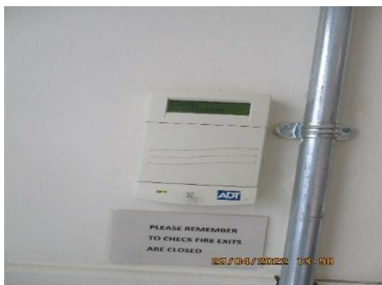
181. Intruder alarm system keypad. Main entrance 1/1
