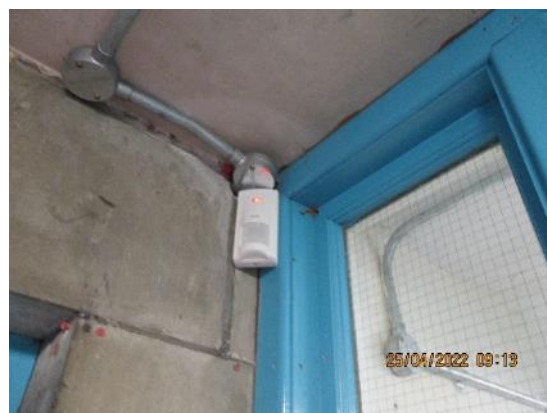
182. Intruder alarm system PIR sensor. Typical throughout.
