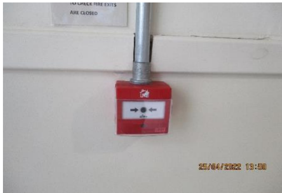
173. Fire alarm break glass call point – typical.
