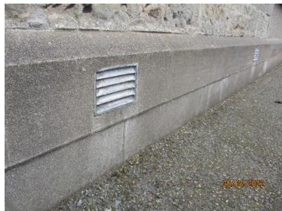
42. Main school, underfloor ventilation
