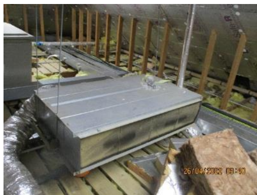
202. Air conditioning unit – indoor. Serves kitchen 1/42.
