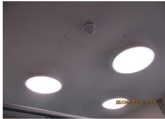
208. Lighting – dining block girls toilets. 1/51
