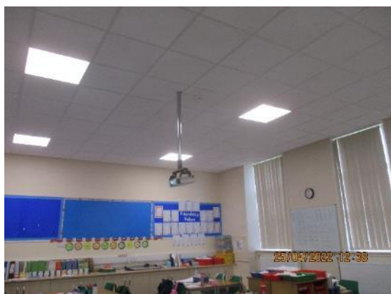
165. Lighting – typical classroom
