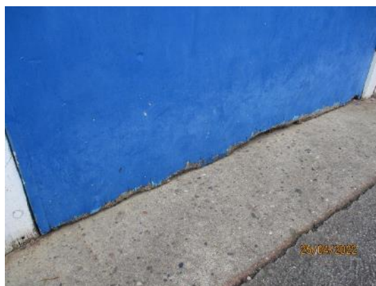
50. Timber wet rot
