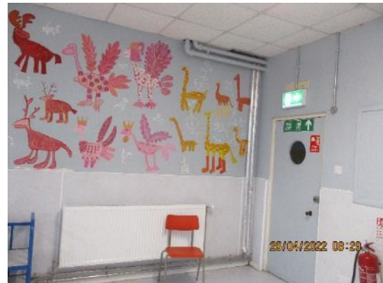
198. Radiator – typical dining hall.
