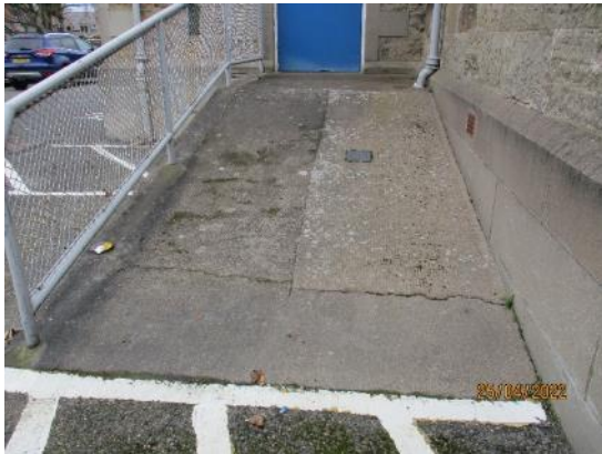
74. Cracked concrete ramps
