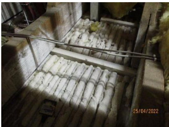
21. Insulation missing in main school roof
