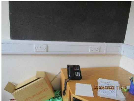
161. Plastic dado trunking and sockets and switches. Typical classroom.
