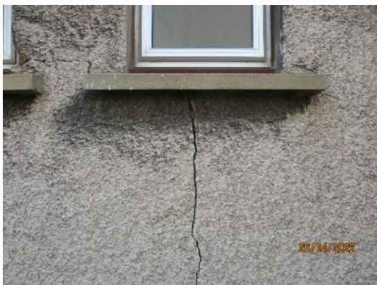
41. Cracking to Dining Hall walls
