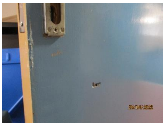
113. Damaged timber doors
