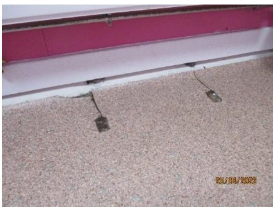
78. Holes in sheet vinyl
