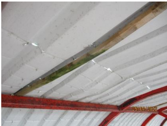
245. Damage to the profile cladding
