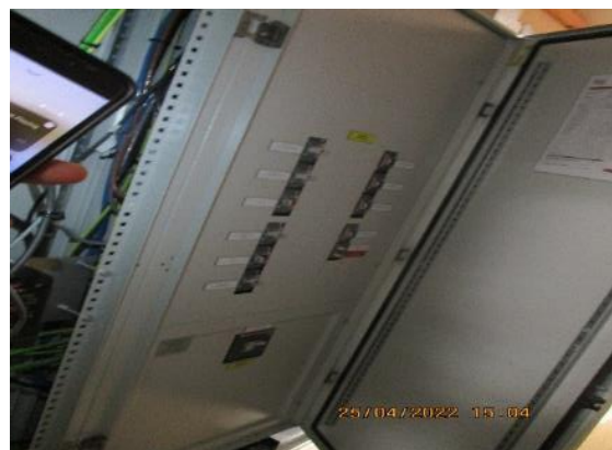
158. Main panel distribution power board 1-16 cupboard.
