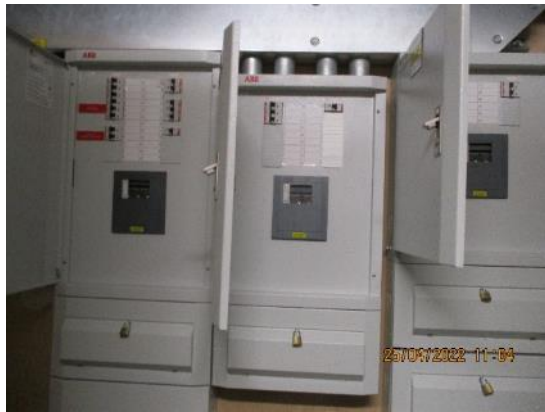
159. Distribution boards. Lighting and power typical.
