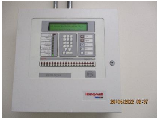
171. Fire alarm control panel main entrance 1/1
