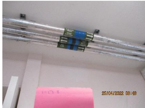
150. Pipework – hot water distribution.
