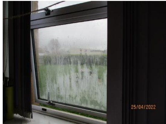
58. Defective double glazed units
