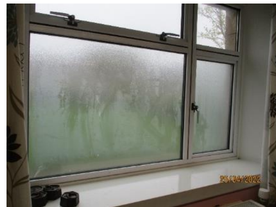
60. Defective double glazed units
