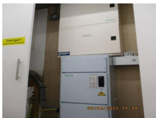
206. Main switch and distribution board – power. 1/40.
