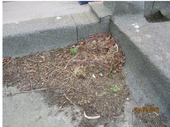
10. Vegetation and debris on flat roofs
