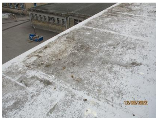
17. Soiled surface of single ply membrane
