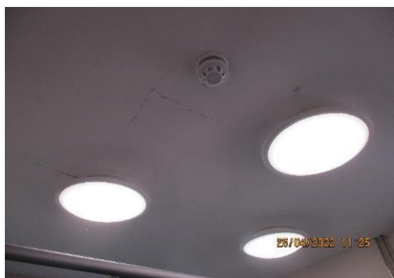
167. Lighting toilets and stores
