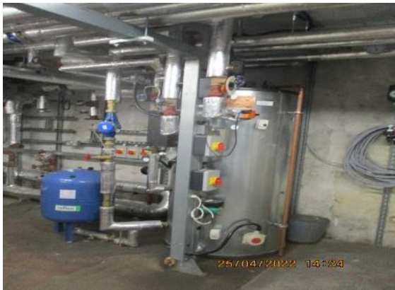
149. Hot water storage calorifier and pipework. 0/1.
