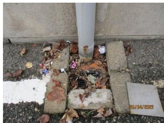
242. Back inlet gullies, partially blocked
