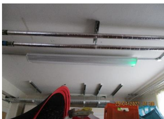
169. Emergency lighting – self - contained non maintained fitting.
