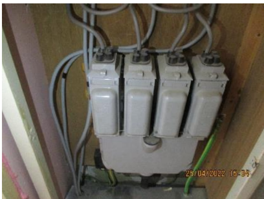
157. Incoming electrical supply and fuses 1-16 cupboard.
