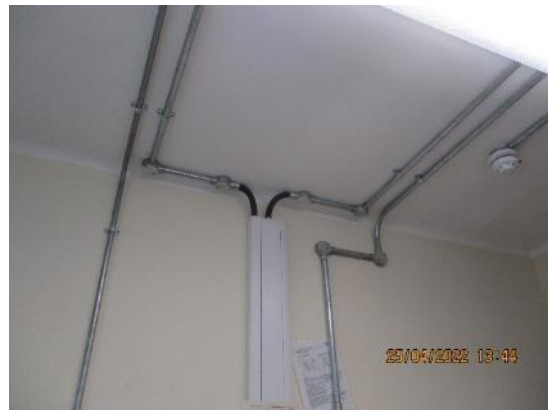
162. Galvanised conduit and distribution general wiring. Typical.
