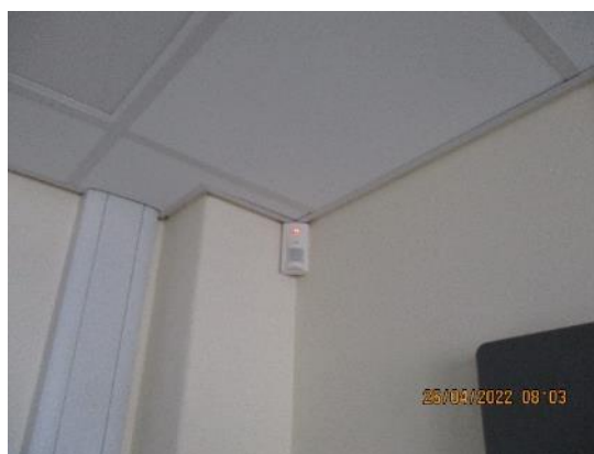
218. Intruder alarm sensor – dining block typical.
