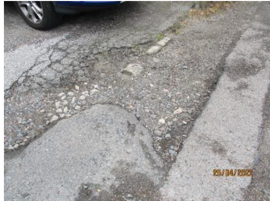
220. Surface breaking up and potholed
