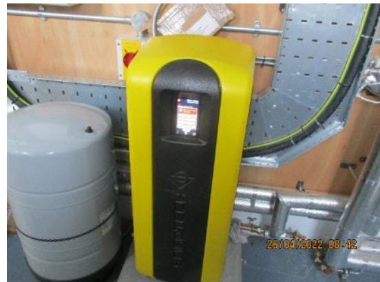
192. Spirovent fill and degas unit plant room 1-50
