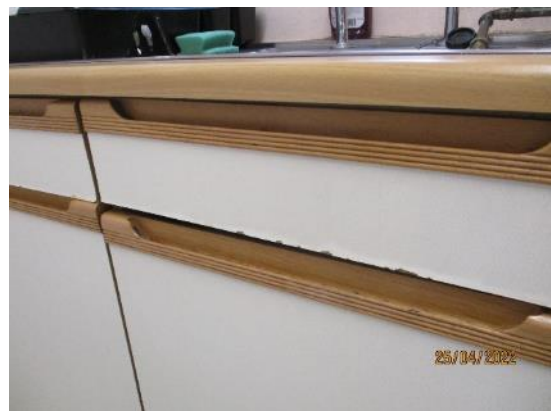
130. Damage to base units
