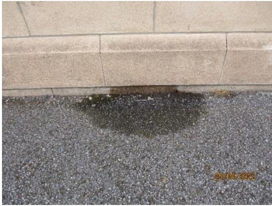
25. Leaking gutter joints
