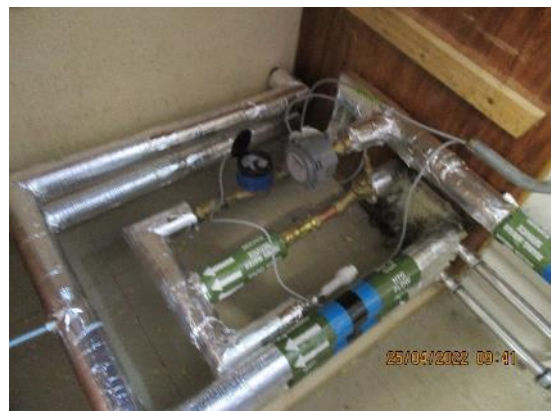
152. Cold water copper pipework and meter. 1/20 box.
