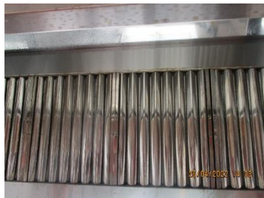
216. Steam oven extract canopy baffles. Detail.
