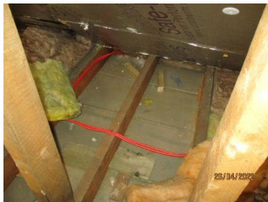
22. Insulation missing in Dining Hall roof
