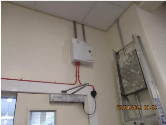
189. Door access control. Magnetic hold open devices complete with fire alarm interface.
