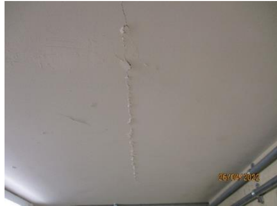
96. Failed taped joints
