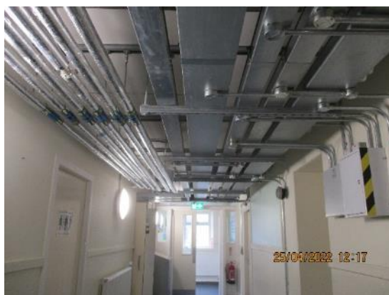
163. Electrical containment for distribution wiring.
