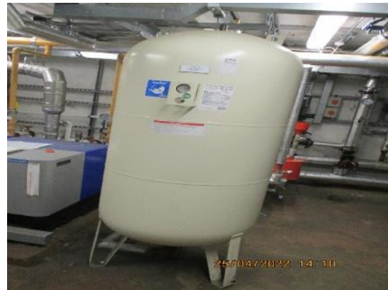
148. Expansion vessel – heating system. 0/1 Boilerhouse.
