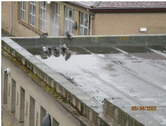
13. Ponding on flat roofs
