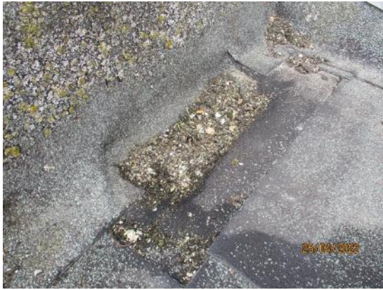
31. Blocked outlets to felt roofs
