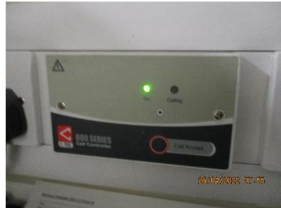
180. Disabled toilet alarm indicator and control unit. Reception office 1/7a.
