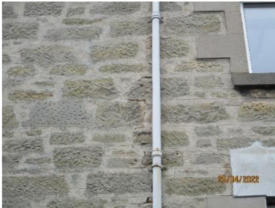
39. Isolated cracking, pointing required
