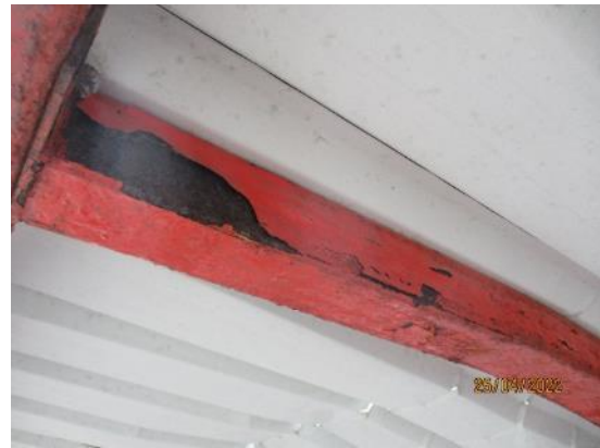
244. Corrosion of the steel frame
