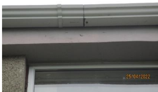
24. Leaking gutter joints
