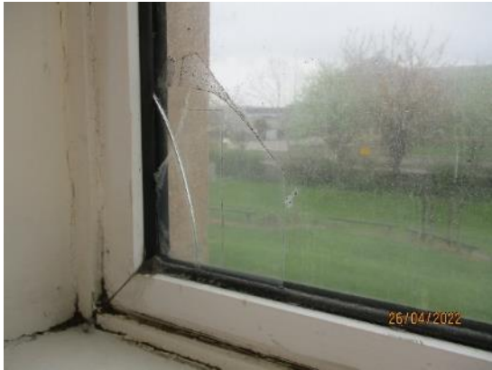
61. Cracked double glazing
