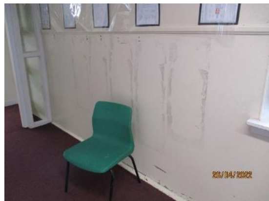
100. Damaged fibreboard linings
