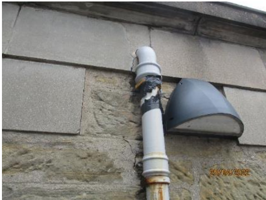
33. Damage to cast iron rainwater downpipes
