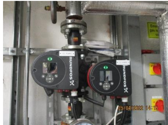
144. Pumps – heating system. 0/1 Boilerhouse.
