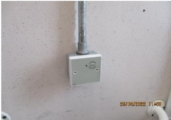
179. Disabled toilet alarm system reset unit. Access shower room 1-30.
