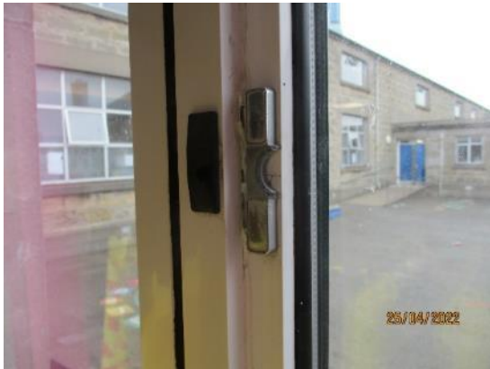
63. Missing ironmongery / sealed windows
