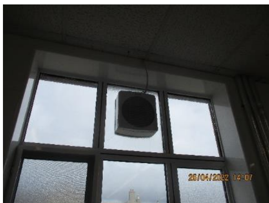
201. Extract fan – kitchen windows. 1-42
