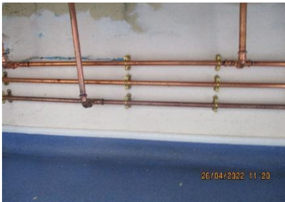
197. Cold water copper pipework – boys toilets 1/52.
