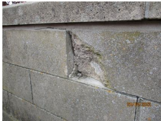
234. Damage to blockwork walls
