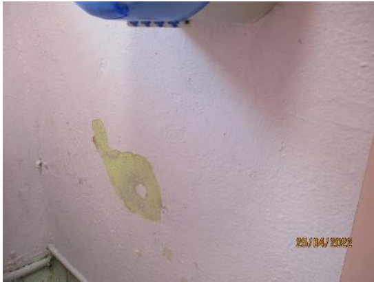
136. Peeling and flaking decoration
