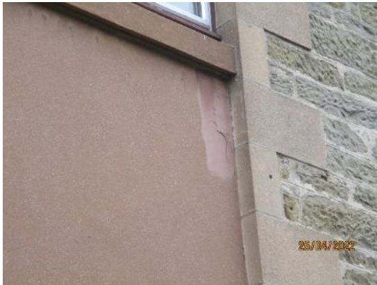
45. Isolated spalling of render panels
