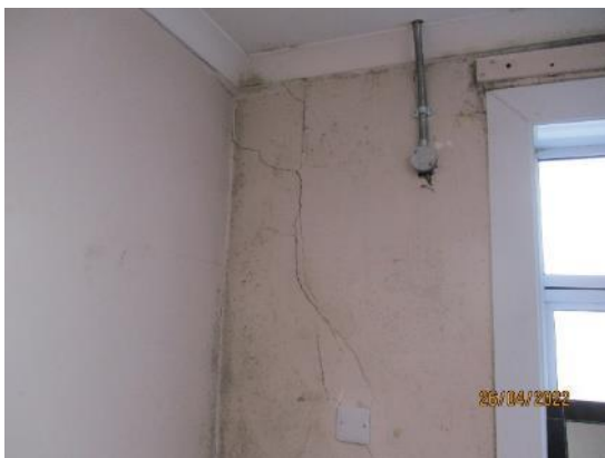
99. Cracking to masonry walls
