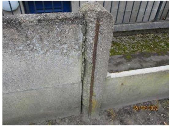
226. Exposed, corroding reinforcement
