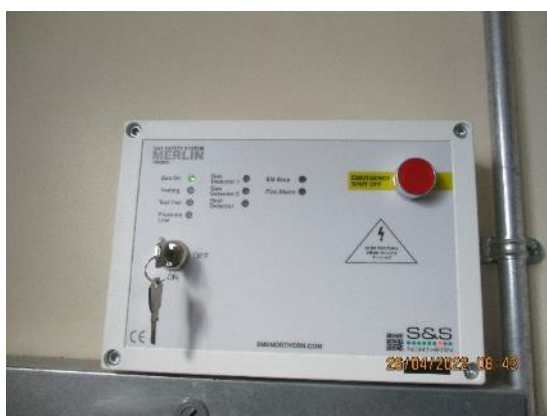
199. Gas safety control panel. Plant room 1/50.
