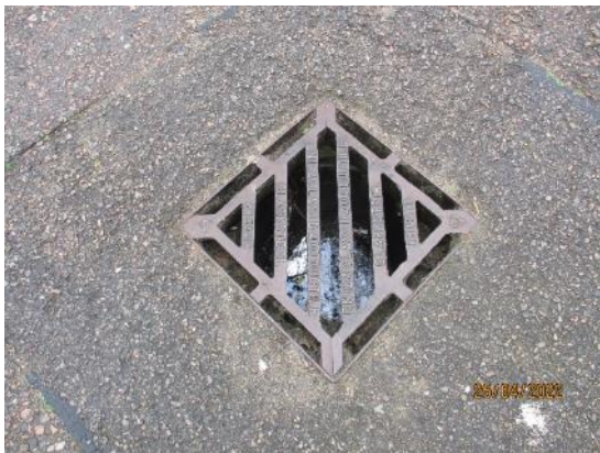
239. Surface water gullies
