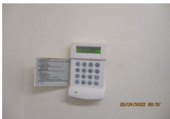
217. Intruder alarm panel 1/47 dining block.
