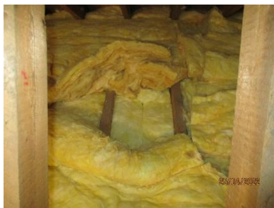
20. Insulation disturbed in main school roof
