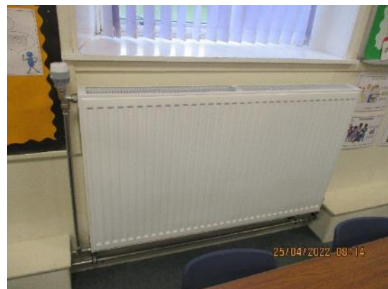
146. Radiator – typical classroom.
