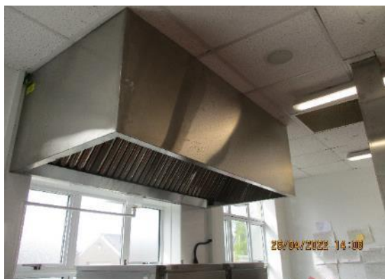
215. Steam oven extract canopy. Main kitchen.
