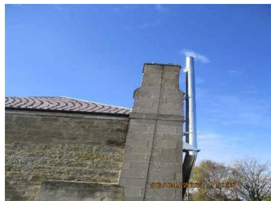
176. Lightning conductor assembly and cable – chimney stack – gym hall 1/5.
