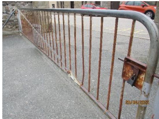
232, Side gate – corrosion and damage
