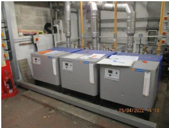
141. Natural gas condensing boilers. 0/1 Boilerhouse.
