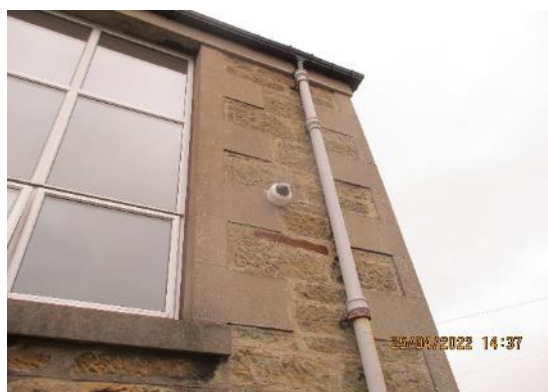
184. CCTV system external fixed camera. Typical.
