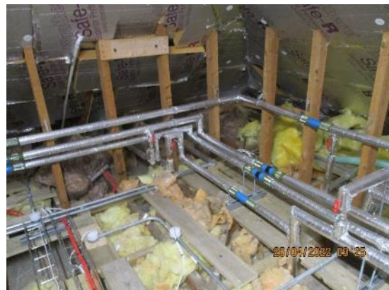
194. Pipework – heating system in attic. Dining block.
