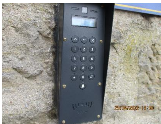
188. Security door access system – main entrance door. Video and audio.
