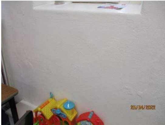
101. Damaged plastered walls
