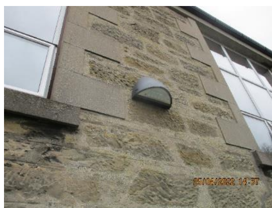
170. Lighting – external building walls.
