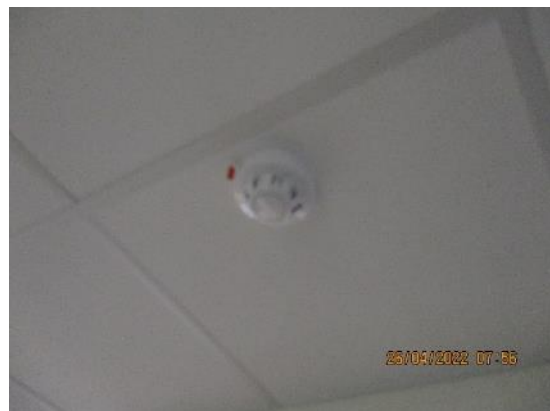
212. Fire detection head dining block typical.
