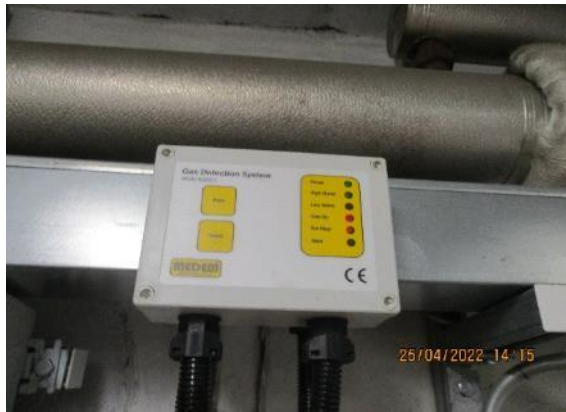
153. Gas safety control panel – plant room 0/1.
