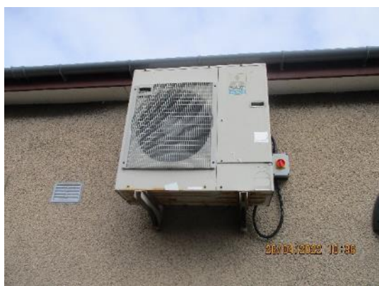
203. Air conditioning outdoor unit. Serves kitchen 1/42
