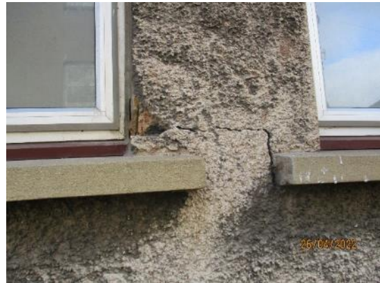
40. Cracking to Dining Hall walls
