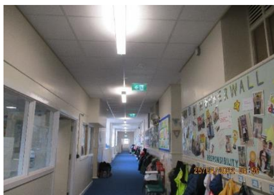
166. Lighting – circulation spaces typical.
