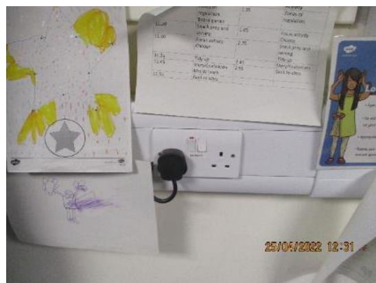
164. Sockets – typical classroom.
