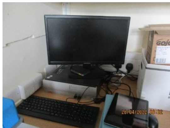
186. CCTV system monitor and recorder office 1/7a
