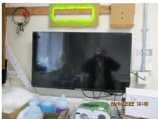
185. CCTV system monitor – janitors room 1/2.
