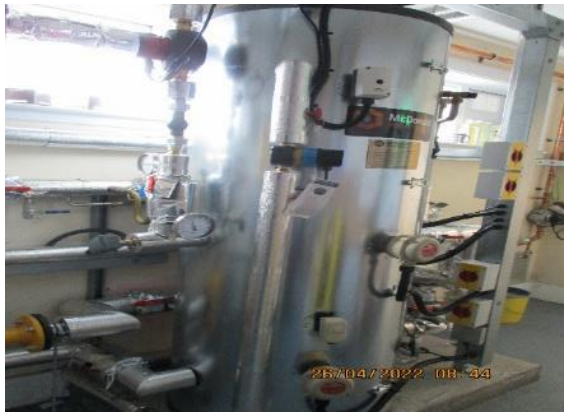
195. Hot water storage calorifier – plant room 1/50
