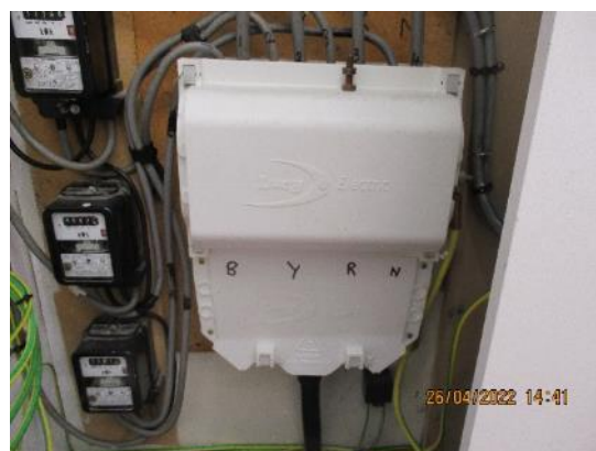
204. Incoming power supply 1/40 kitchen cupboard.
