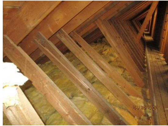
2. Displaced rafter supports
