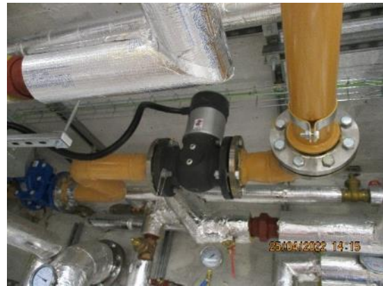
154. Gas pipework and solenoid valve – plant room 0/1.
