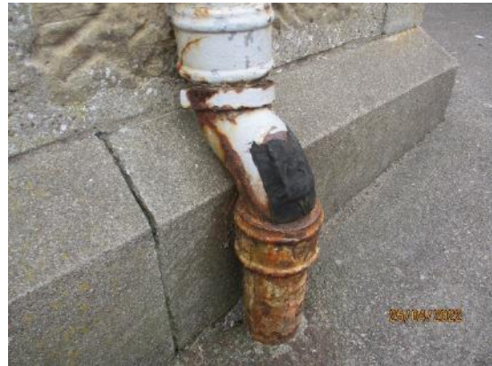
34. Damage to cast iron rainwater downpipes
