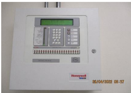
211. Fire alarm panel. Dining block.
