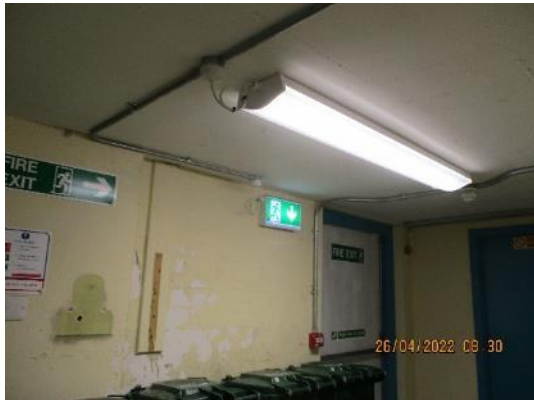
209. Emergency lighting dining block. Typical
