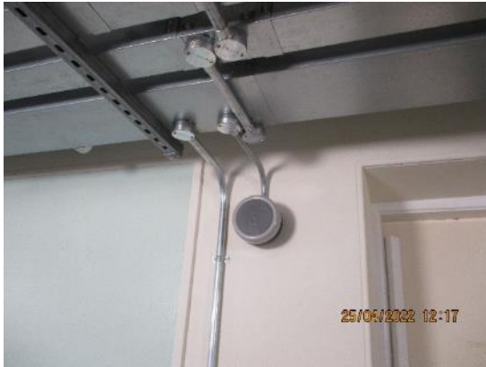
177. Period bell – corridor typical.
