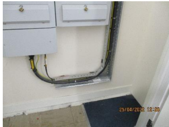
160. Sub mains cabling cupboard 1-22.
