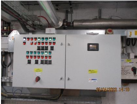
147. BMS control panel – heating, ventilation and electrical. 0/1 Boilerhouse.
