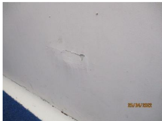
106. Fibreboard linings damaged
