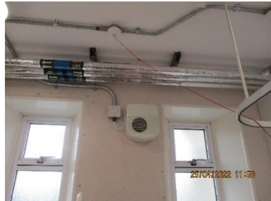
156. Extract fan Access shower room 1-30.
