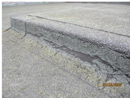
12. Felt surface cracking
