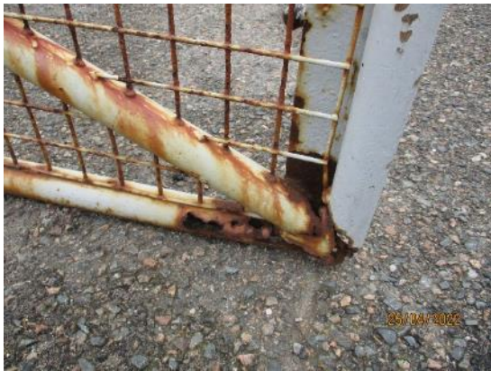
231. Corrosion of tubular gates
