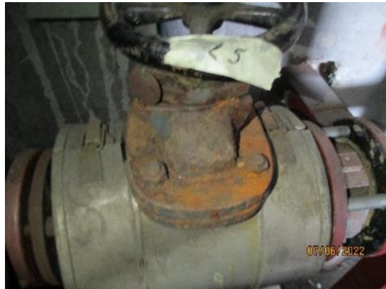
104. Heating system valve – boiler house 1-19
