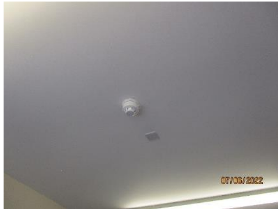
140. Smoke detector head. Typical.
