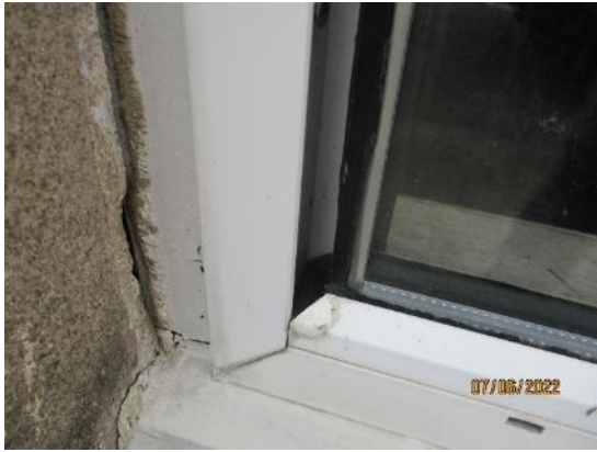
31. Missing glazing bead to boiler room
