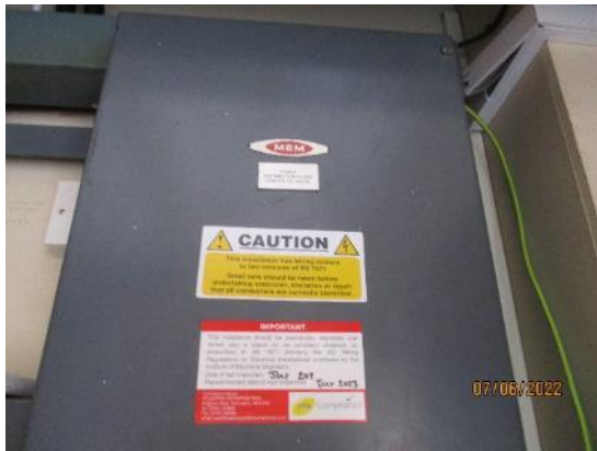
119. Distribution board – power. Store 1/3
