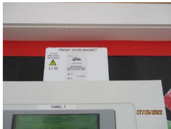
154. Fire alarm security door auto release interface. Entrance hall 1/2.
