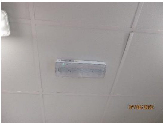
135. Emergency lighting. Typical – kitchen 1/17
