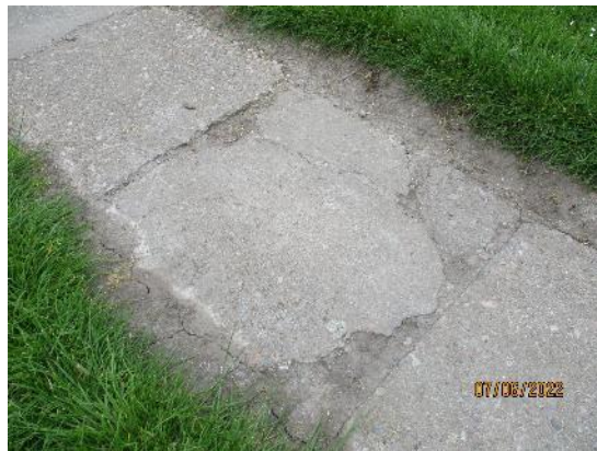
170. Cracked and uneven
