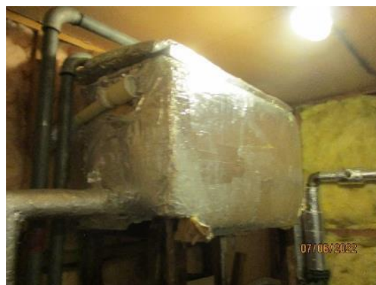
106. Heating system – feed and expansion tank. 1/20
