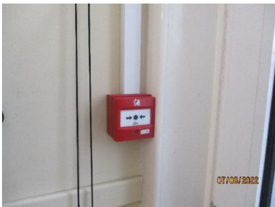
141. Fire alarm call point typical.
