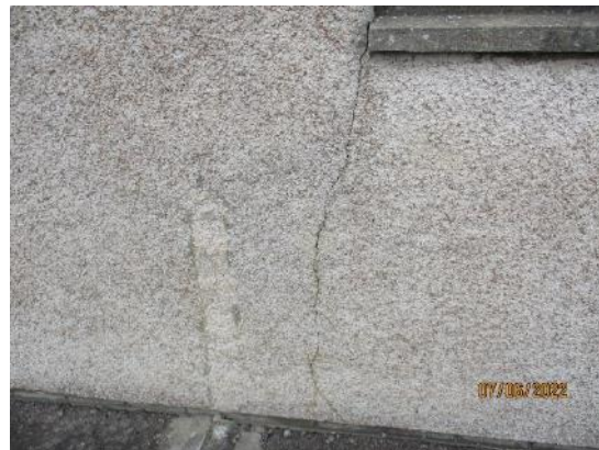
16. Isolated hairline cracking
