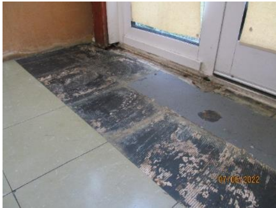
52. Missing vinyl tiles
