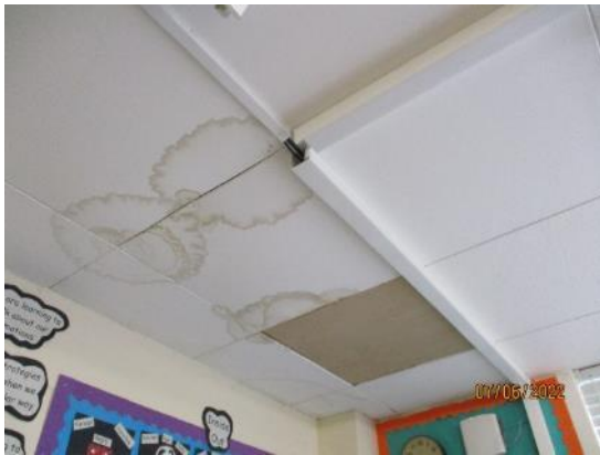
60. Watermarked ceiling tiles to classrooms
