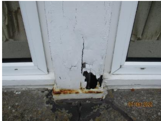
34. Rotten timber frame
