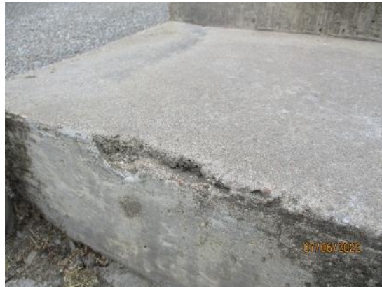
46. Damage to nosings
