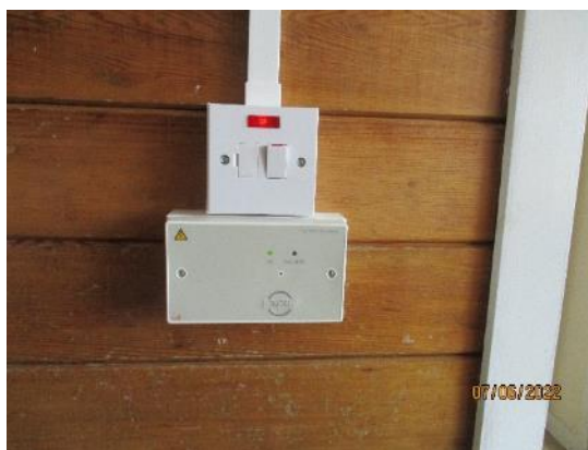
148. Disabled alarm alert unit. Cloakroom 1/9.
