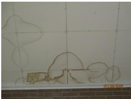
58. Watermarked ceiling tiles
