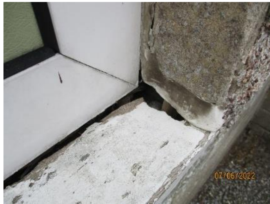
38. Rotten timber sills
