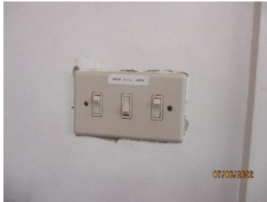
128. Light switch. Kitchen 1/17
