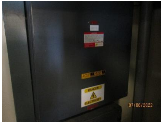
120. Distribution board – kitchen. Store 1-18
