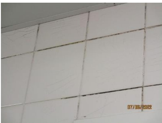
70. Soiled grouting to tiles
