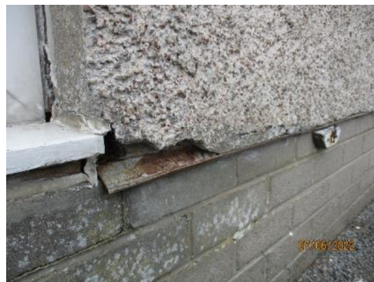
18. Corrosion and damage
