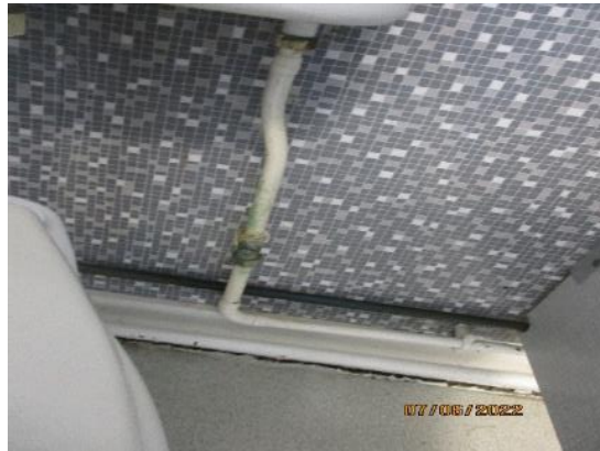
110. Cold water pipework – girls toilets 1-8
