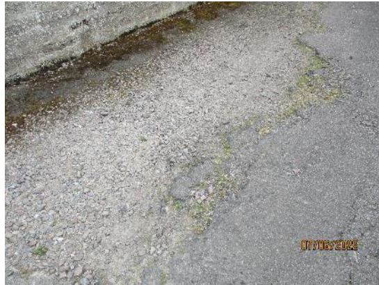
156. Surface erosion and potholes
