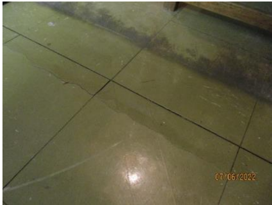
51. Damaged vinyl tiles
