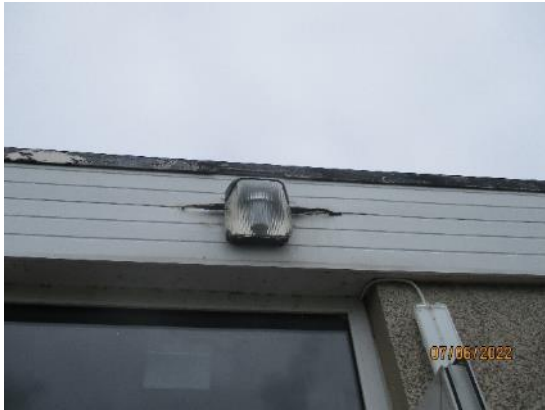
137. External lighting typical.
