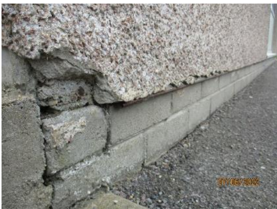
17. Damage to bellcast bead
