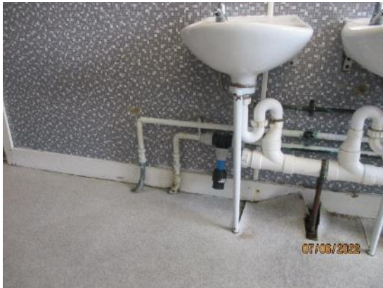
109. Hot water pipework. Girls toilets 1-25
