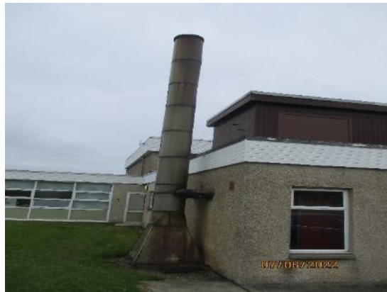
102. Boiler common chimney. 1-19 External.
