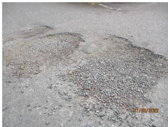
160. Surface erosion and potholes
