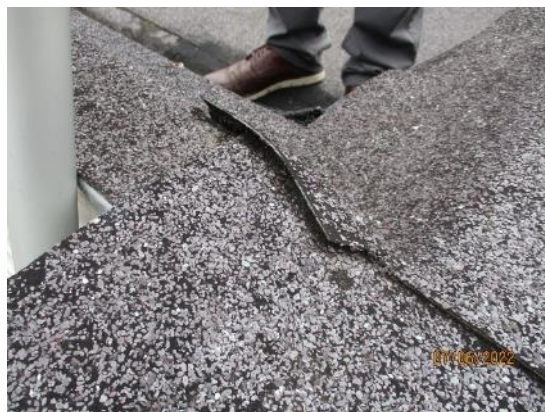
6. Open joints in felt roofing
