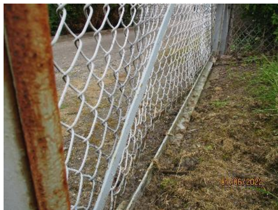
178. Damage and surface corrosion
