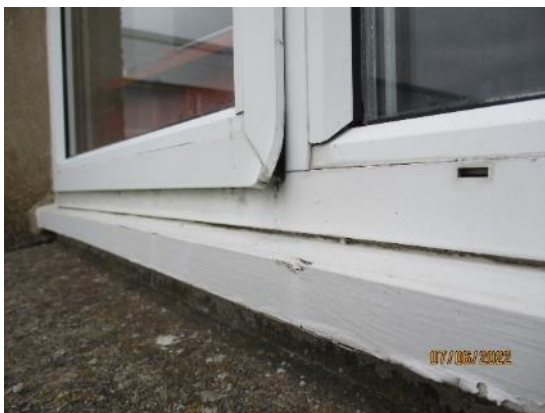
29. Damaged window casement
