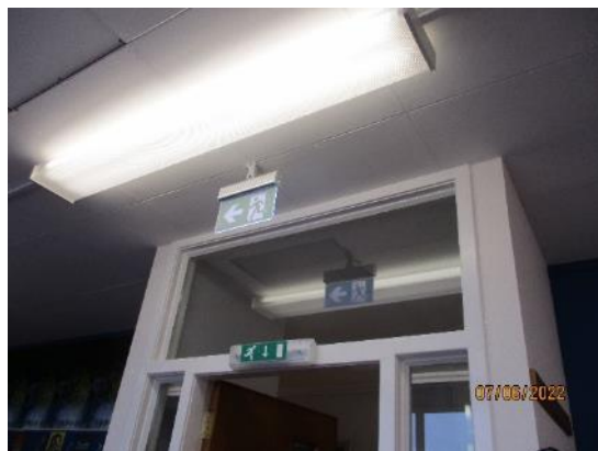
136. Emergency exit sign lights. Typical – library 1/12
