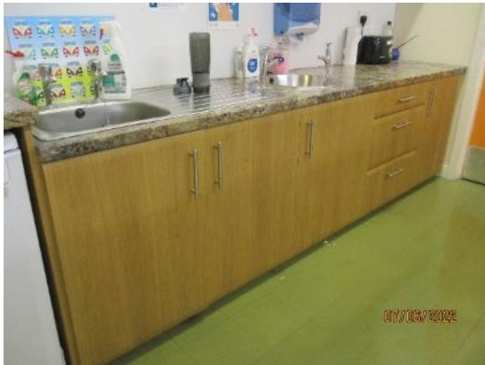
97. Kitchen base units
