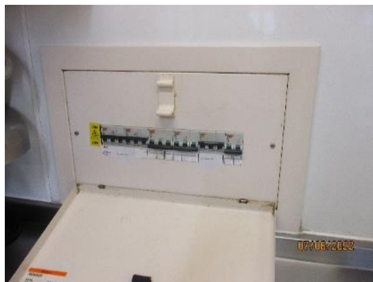
124. Distribution board. Power – kitchen 1/17
