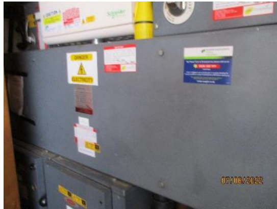
122. Main busbar – store 1/3.
