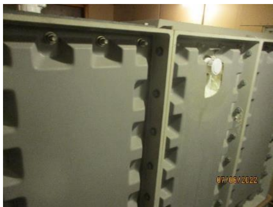
111. Cold water storage tank – tank room 1-20.
