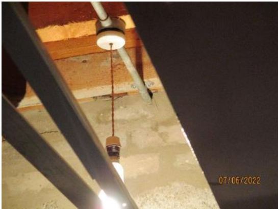
133. Lighting – external store example.
