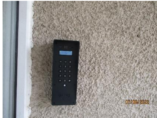
152. Door access security system keypad and camera unit. Main entrance.
