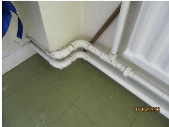
108. Heating system pipework. Typical
