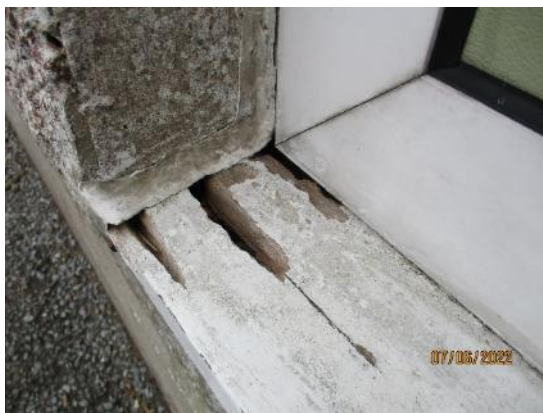
36. Rotten timber sills
