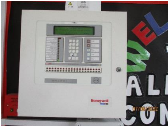
139. Fire alarm system control panel. Entrance hall 1/2
