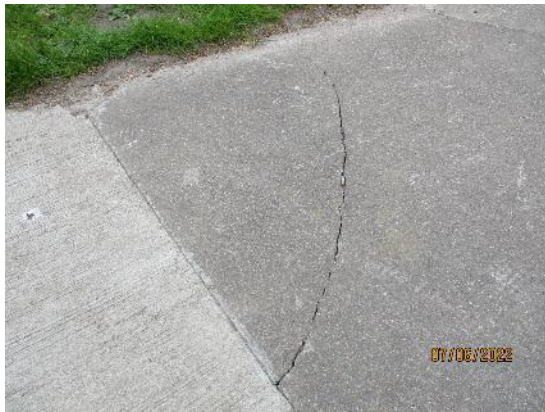
167. Cracked concrete paths
