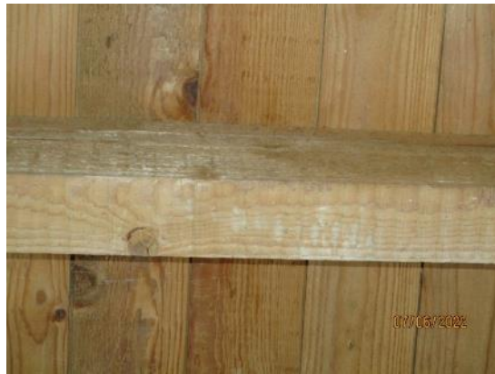
2. Woodworm in joists
