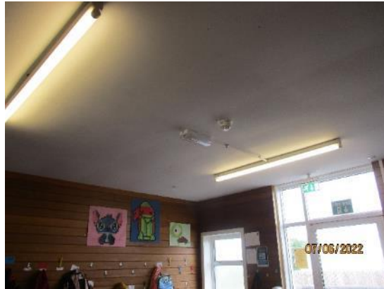
132. Lighting – cloakroom example.
