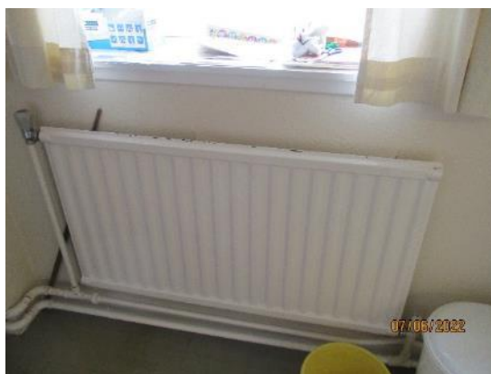
105. Radiator – steel panel. Heating system typical.
