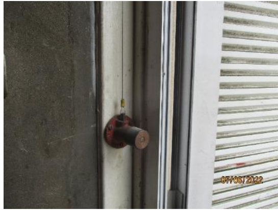
114. Oil safety push button cut off system.
