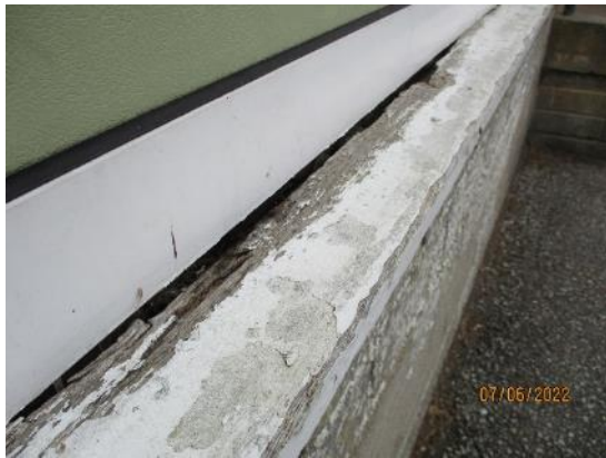
37. Rot and missing sealant
