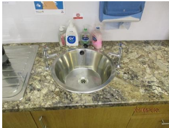
90. Stainless steel hand washing sinks
