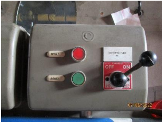
107. Heating control switches. Boiler house 1-19
