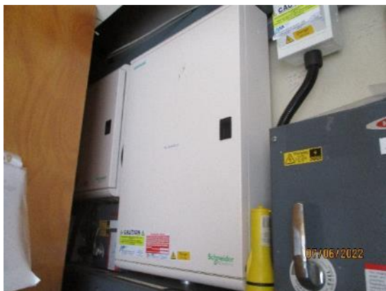
123. Distribution board power. LP1 – Store 1/3
