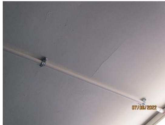
61. Plasterboard with hairline cracking
