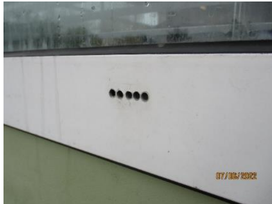
28. Missing weep hole covers
