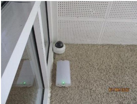
149. CCTV fixed camera. Main entrance.
