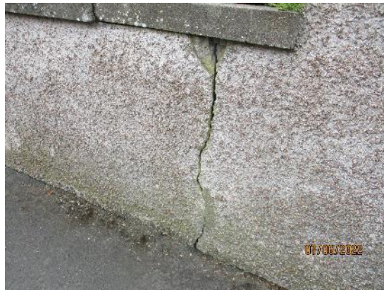
180. Cracks in boundary wall
