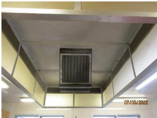
117. Kitchen extract canopy and filter unit.
