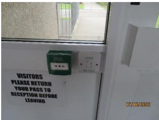
153. Door access system emergency release devices.
