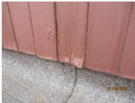
20. Rot in timber boards
