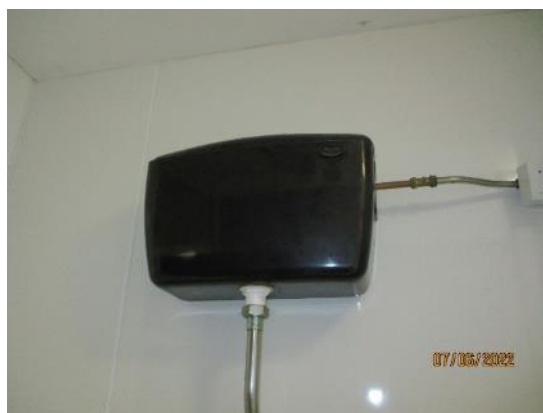
82. High level composite cistern
