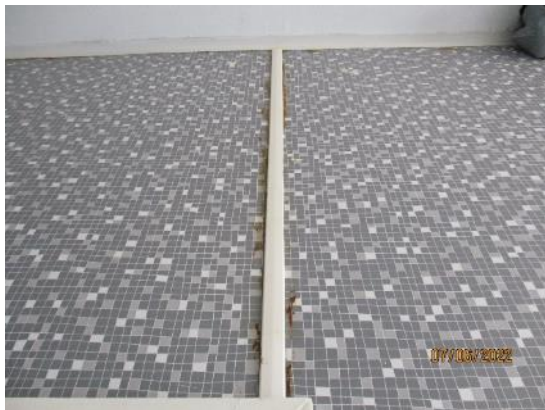
68. Soiled wetwall joints
