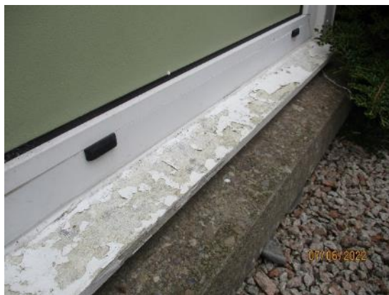
35. Paint peeling on sills
