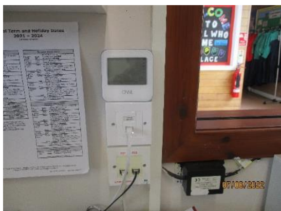
145. Phone outlet sockets – office 1/30
