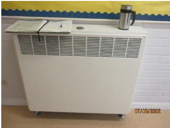
103. Convector heater – heating system typical.
