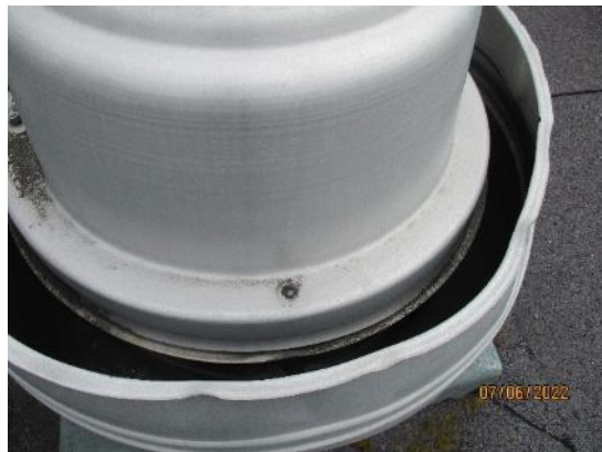
118. Kitchen island extract fan and terminal.
