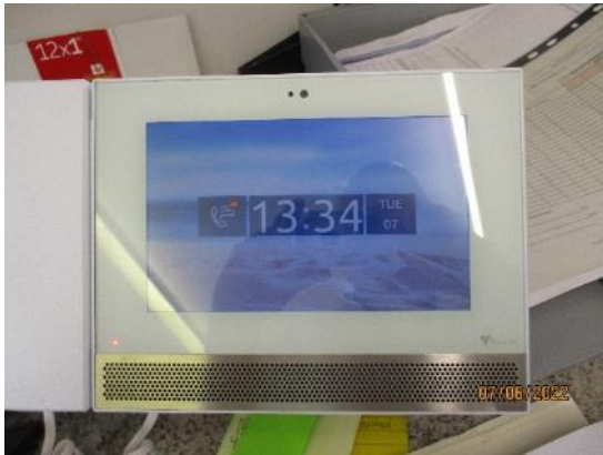
151. Door access security system. Viewer and handset. Office 1/30.
