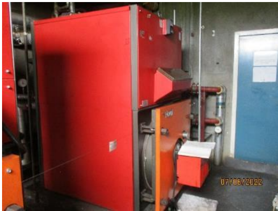
101. Oil shell and tube boiler. Boilerhouse 1/19
