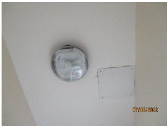
130. Lighting – typical toilet.
