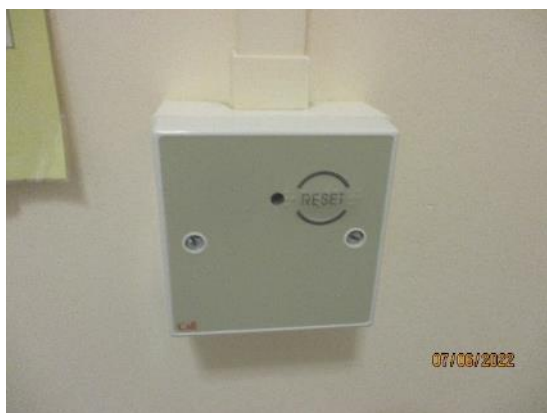
147. Disabled alarm reset unit. 1/8a Access WC
