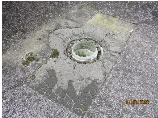
10. Cracking of surface
