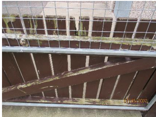
176. Timber rot and flaking paint
