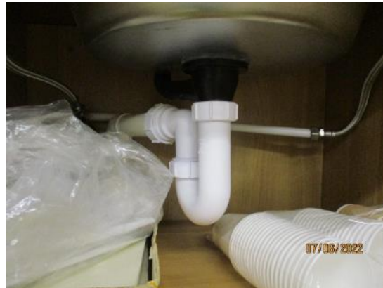
92. PVC waste pipes
