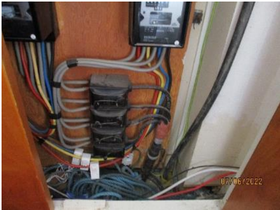
121. Incoming power supply and main fuses. Store 1/3
