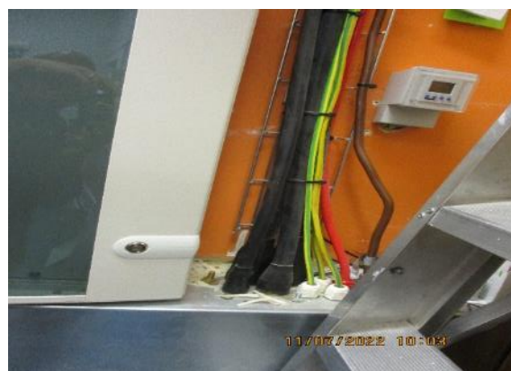
160. Sub mains cabling cupboard 1-31
