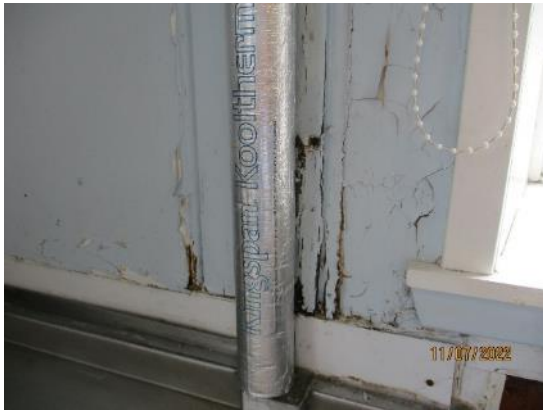
92. Damage to lath & plaster walls
