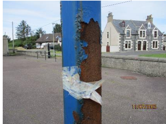
218. Steel stands with surface corrosion
