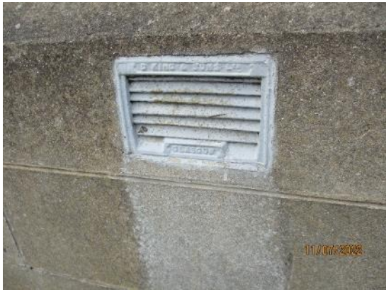
32. Under floor ventilation
