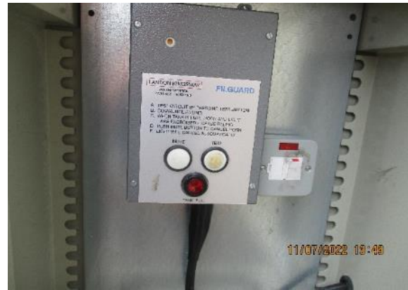
150. Oil tank overfill alarm device – external.
