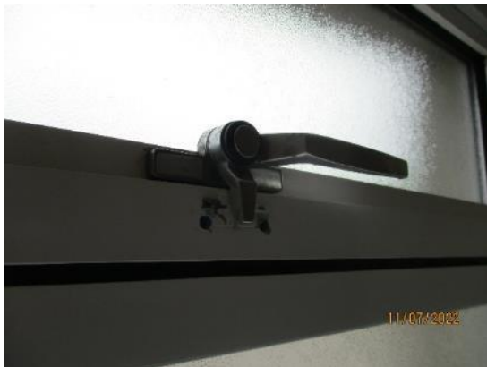
50. Window handles and missing friction wedges
