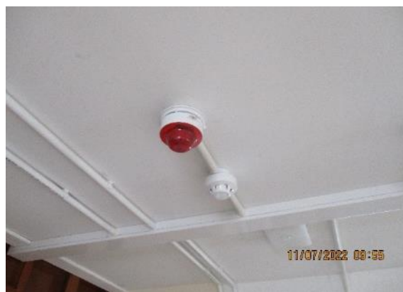
174. Fire alarm smoke detector and strobe. Typical.
