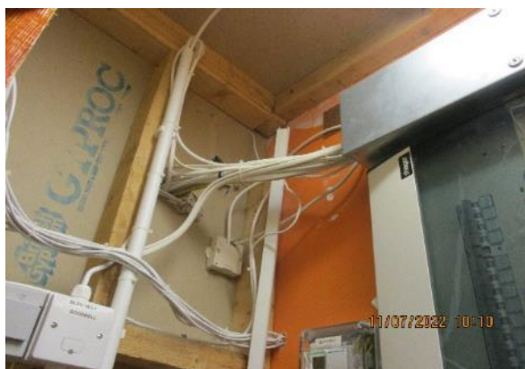
159. General wiring 1-31 cupboard
