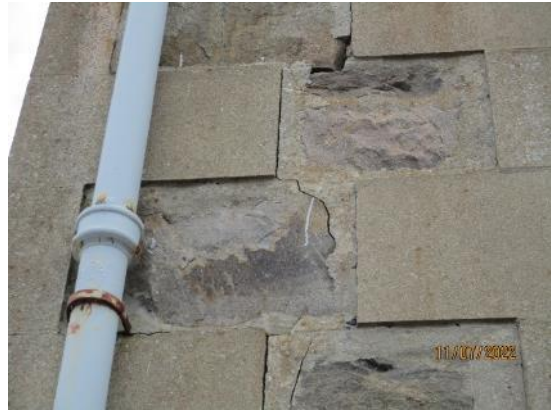
31. Cracking at corner stones
