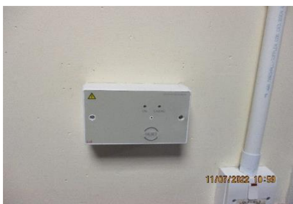
177. Disabled alarm system alert unit. 1/13 for WC 1/17a
