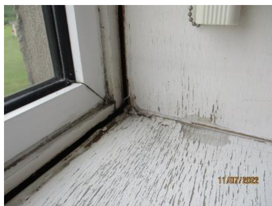
45. Gap between windows and internal frame
