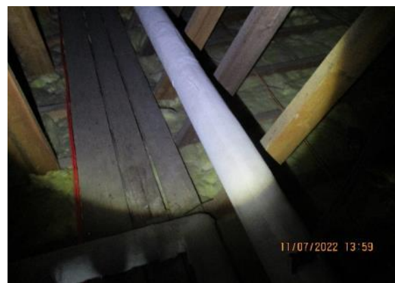
142. Heating pipework – attic space.
