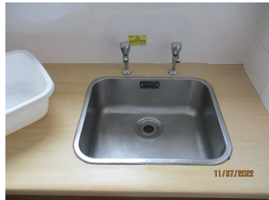
129. Stainless steel inset classroom sinks
