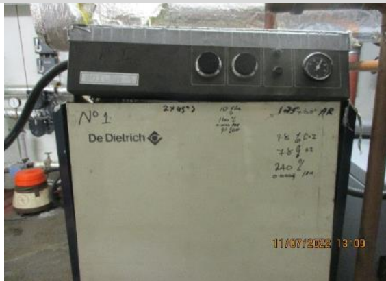
137. Oil Boiler no.1 – Basement boilerhouse 0-41
