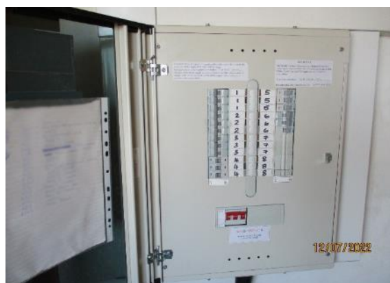
158. DB – GLP3 – Cupboard 2-32
