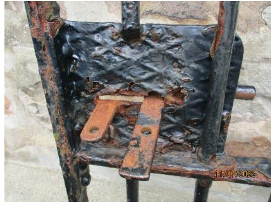
200. Extensive penetrating corrosion
