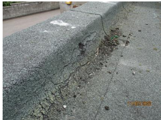
10. Cracking and blistering
