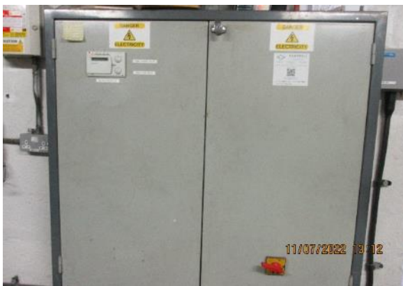
147. Heating control panel – boilerhouse 0/41
