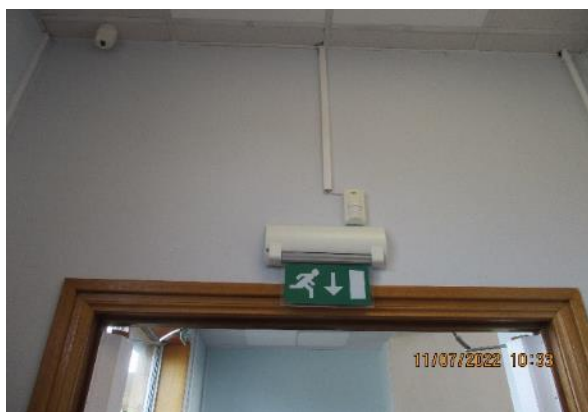
167. Emergency exit escape route sign light. Typical.
