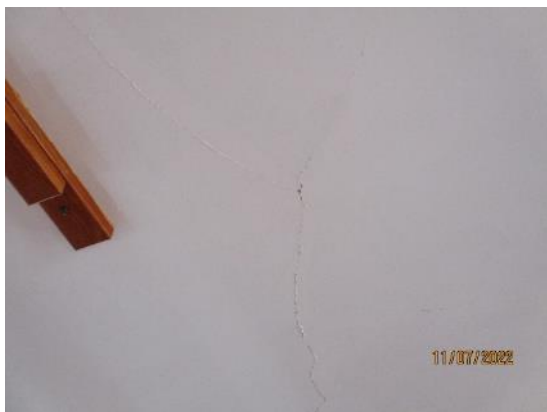
86. Cracked lath & plaster ceilings
