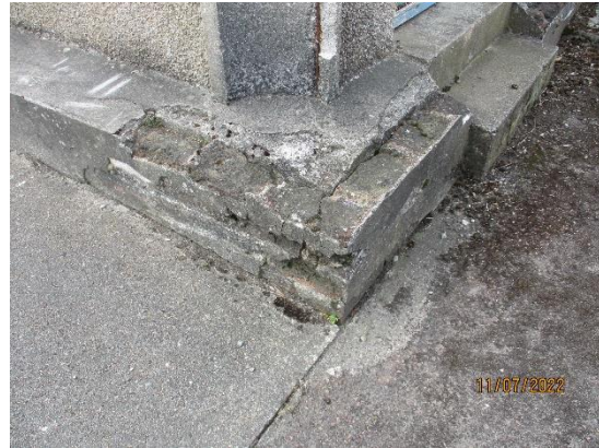
212. Brick plinth, breaking up
