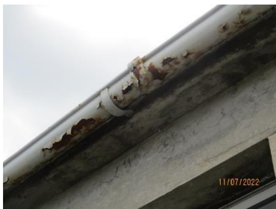
17. Extensive surface corrosion
