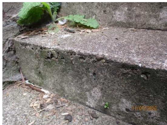
59. Minor surface erosion
