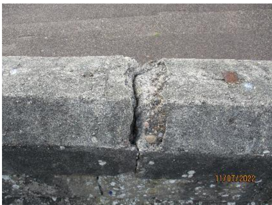
203. Damage to concrete coping
