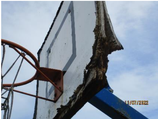
219. Backboards laminating and crumbling
