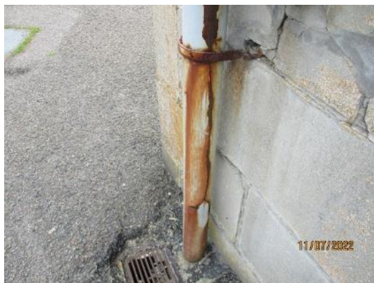
22. Cracked and leaking cast iron downpipes
