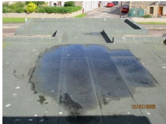
8. Ponding following overnight rain
