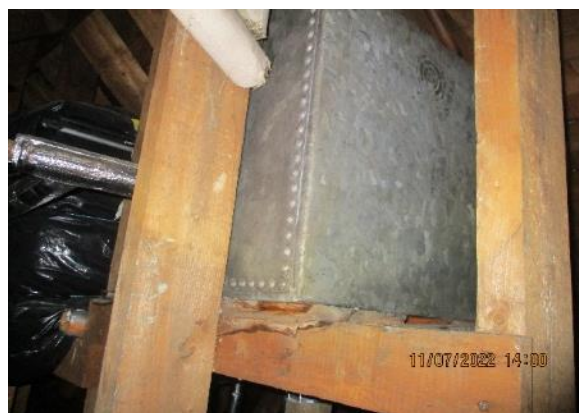
141. Heating system feed and expansion tank. Attic.
