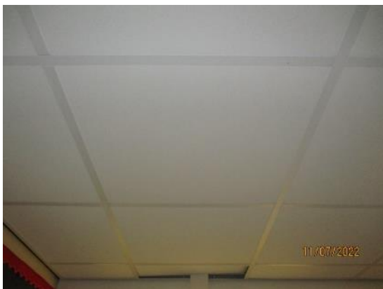
82. Suspended ceiling tiles
