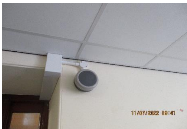
175. Period bell – corridor 1/2. Typical.
