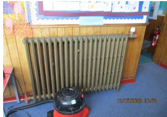
144. Radiator – heating system typical.
