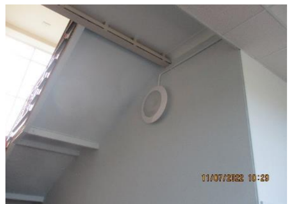
166. Lighting under staircase typical.
