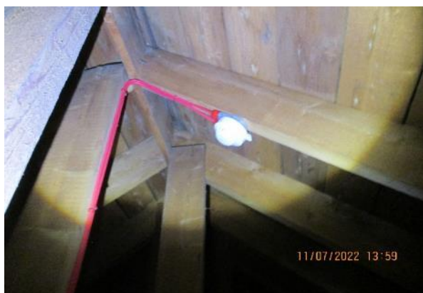
173. Fire alarm wiring and smoke detector. Attic.
