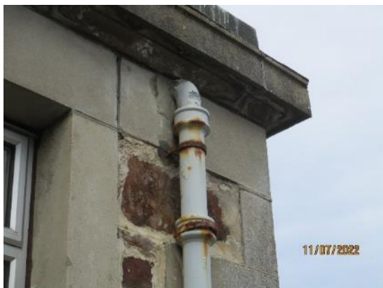
21. Corrosion to cast iron downpipes
