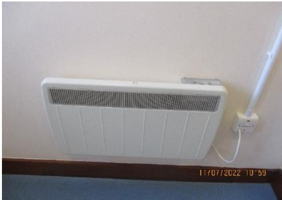
145. Electrical Convactor heater – Girls toilet. 1/8
