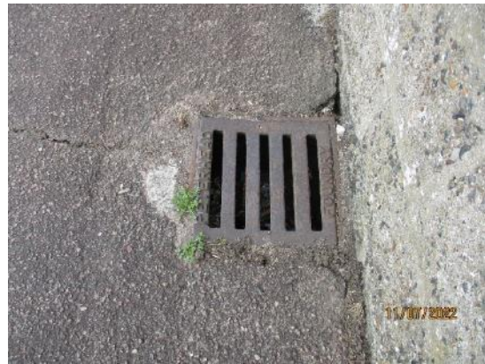
206. Surface water drainage
