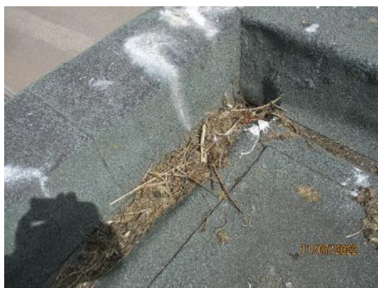
20. Outlets blocked with nesting material
