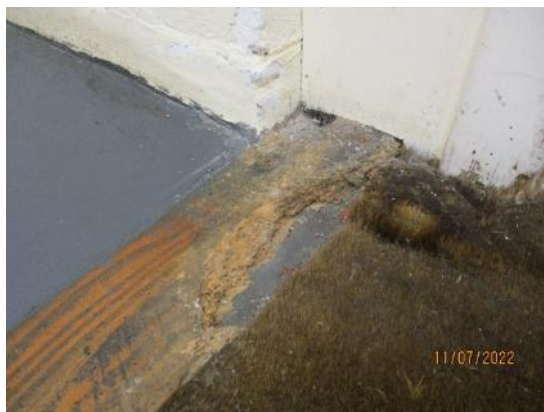
75. Extensive woodworm damage
