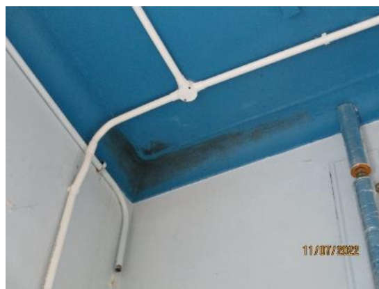
85. Lath & plaster ceilings with mould growth
