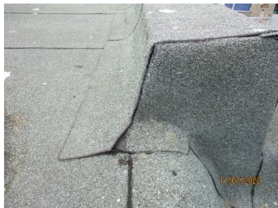
6. Open joints in felt roofing
