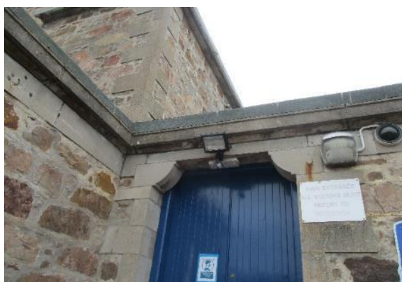
169. External lighting. Bulkhead and flood. Main entrance
