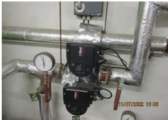
139. Pumps – Primary boilerhouse 0/41
