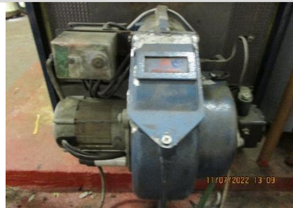
138. Boiler no.1 Burner assembly
