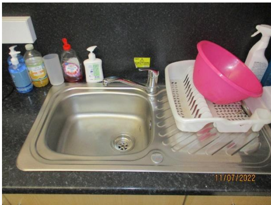
128. Stainless steel classroom sinks
