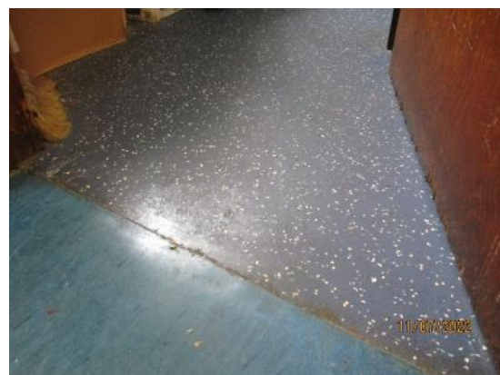
65. Sheet vinyl flooring, worn
