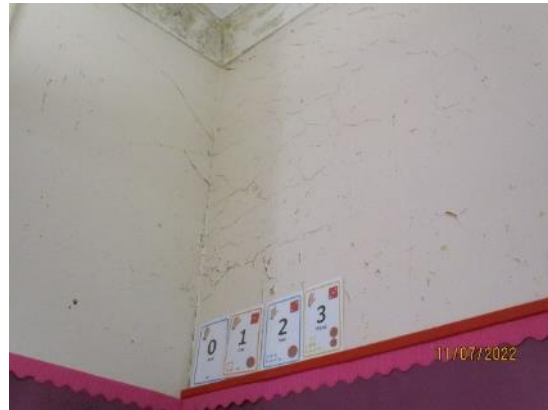
93. Damp plastered walls
