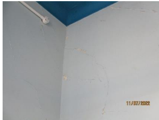
91. Cracking to lath & plaster walls
