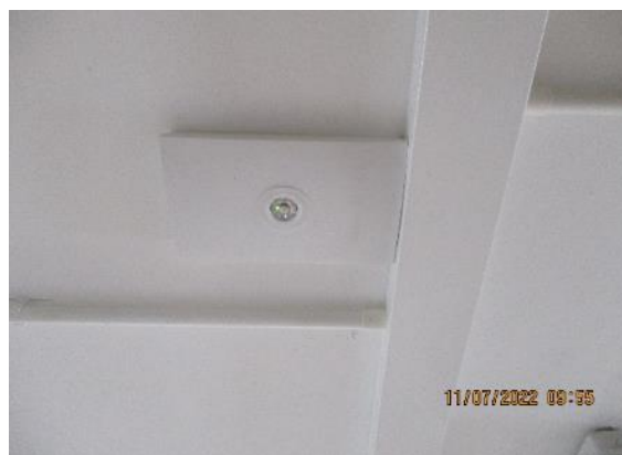
168. Emergency lighting self-contained unit. Typical.
