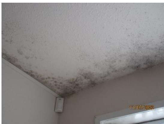
84. Plastered ceilings with mould growth
