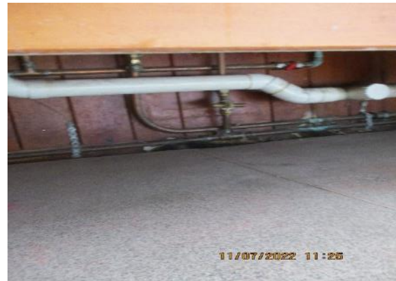
152. Pipework – hot water class 1/25.
