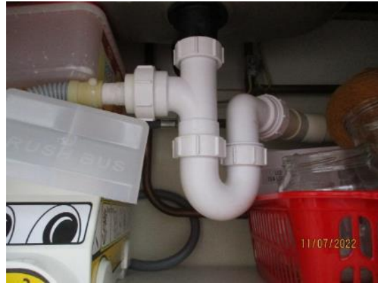
133. UPVC waste pipes
