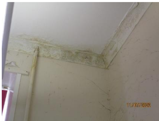
87. Damp ceiling and cornice
