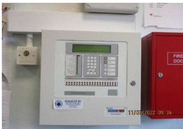
171. Fire alarm control panel. 1/2 corridor.
