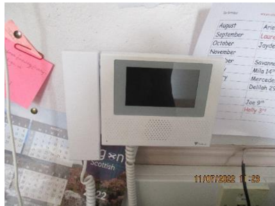
182. Door entry control system handset and viewer. 1/25 and reception office.
