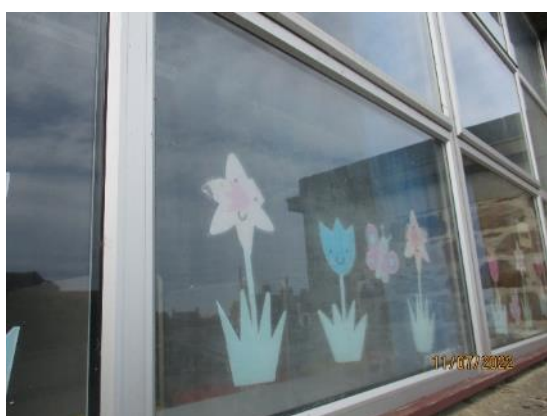
46. Fogged double glazing units
