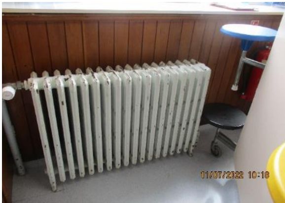
143. Radiator – heating system. Kitchen / cast iron.
