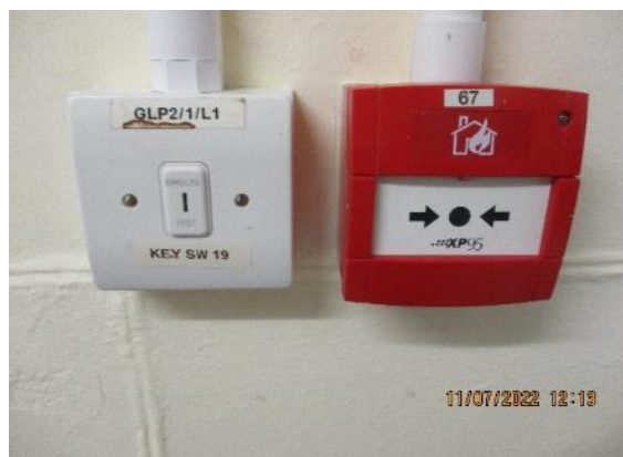
172. Fire alarm call point. Typical.
