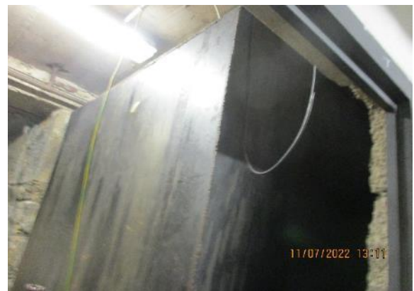
148. Oil storage tank – boilerhouse 0/41
