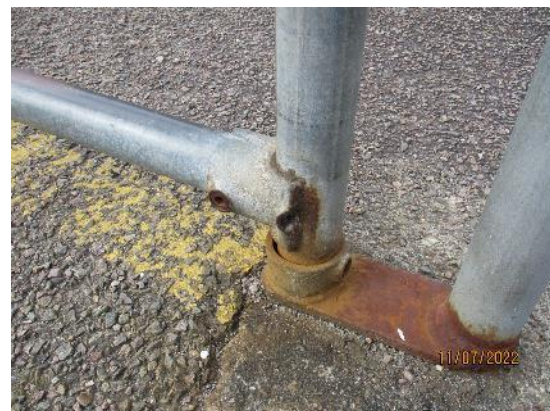
196. Surface corrosion and damage
