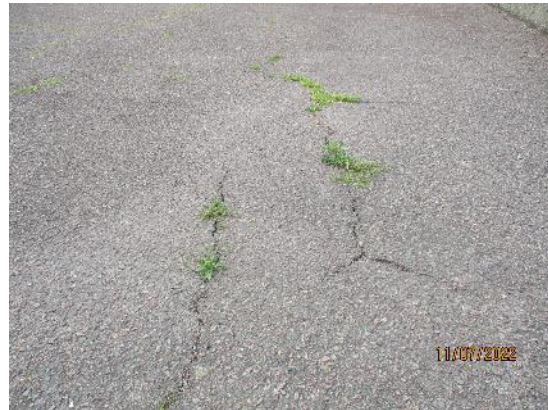
188. Surface cracking and vegetation
