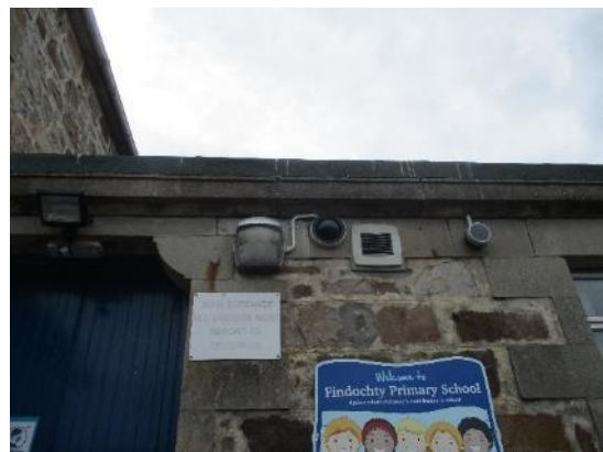
184. CCTV camera. Main entrance.
