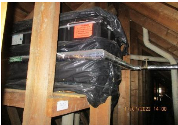
153. Cold water storage tank. Attic.
