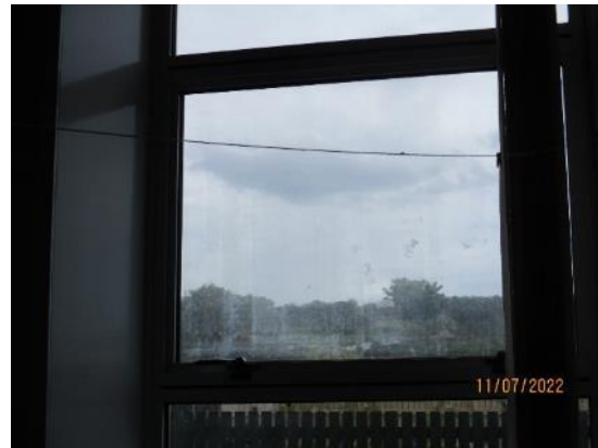
49. Fogged double glazing
