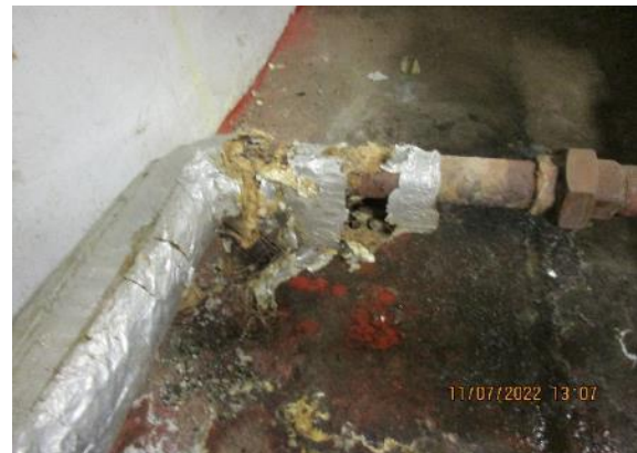
140. Pipework – Heating system boilerhouse 0/41
