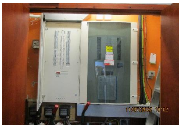
157. Main switchboard and DB GLP1 – cupboard 1-31
