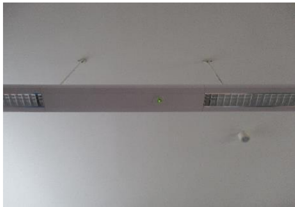
163. Lighting – typical classroom.
