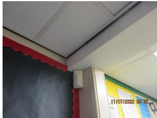
180. Intruder alarm system PIR corridor 1/2 Typical.
