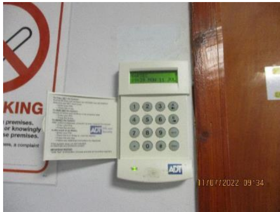
179. Intruder alarm system key pad corridor 1/2.
