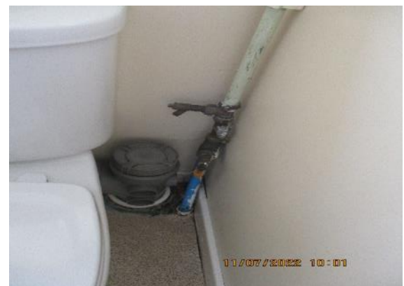
154. Cold water supply pipework. Girls toilet 1/8
