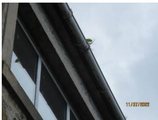
18. Vegetation in gutters
