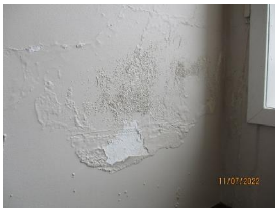
94. Damp to plastered walls
