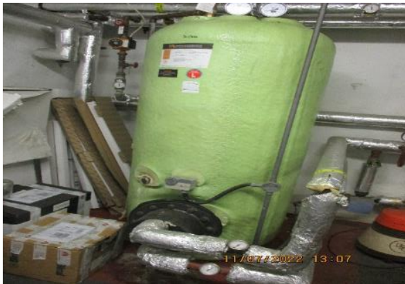
151. Hot water storage calorifier. Boilerhouse 0/41
