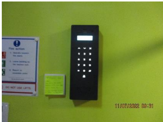
181. Door entry control system video and audio unit. Main entrance and West entrances.
