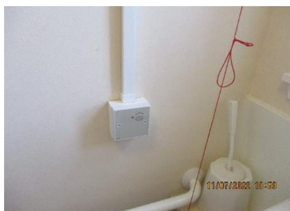
178. Disabled alarm system pull chord and reset – 1/17a
