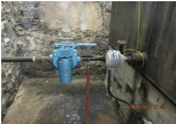
149. Oil pipework and control devices. Boilerhouse 0/41
