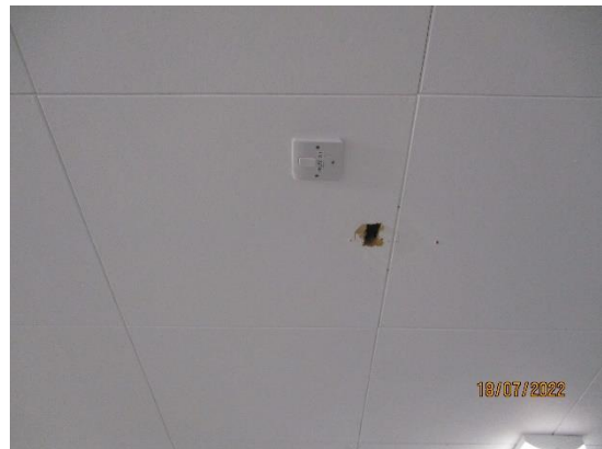
68. Damaged fibre tiles
