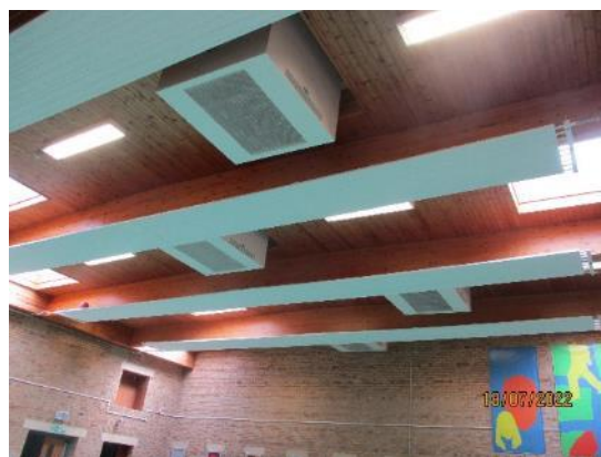
155. Automatic Ventilation Units. Hall ceiling mounted.
