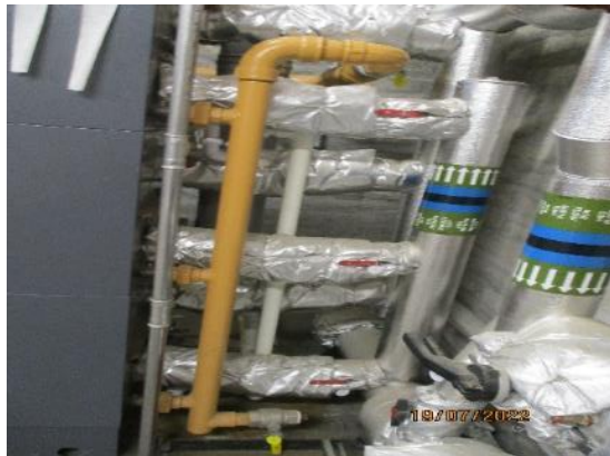
144. Gas supply pipework to modular boilers.
