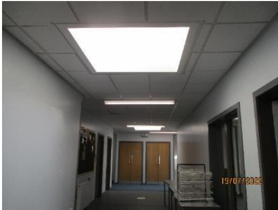
166. Lighting – main school corridor.
