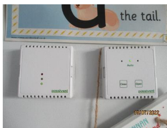
153. Passivent controls. Modular classrooms. Typical.
