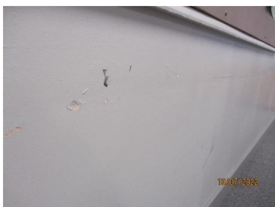
80. Damage to plasterboard
