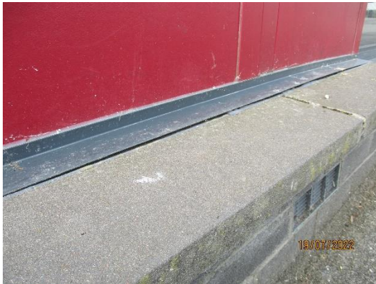
27. Poor sill detail
