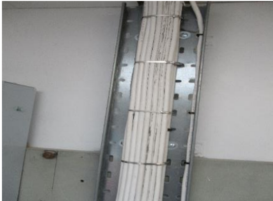
162. General wiring – circuit distribution. Switch room.
