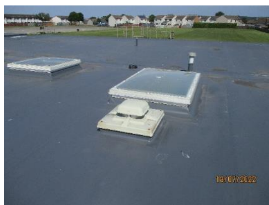
149. Extract fan terminations. Main roof.
