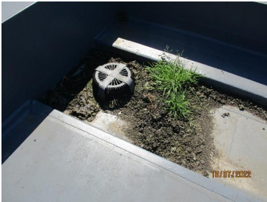
15. Partially blocked gutters
