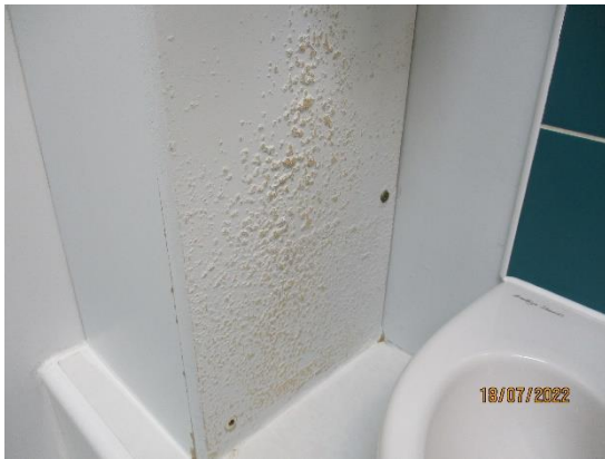
110. Blistering paint to pipe boxes
