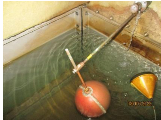
139. Cold water storage tank – above hall cupboard.
