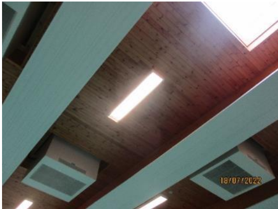
132. Roof mounted radiant panels. Heating – hall.
