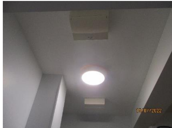
169. Lighting – main school store.
