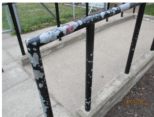
42. Peeling paint to guardrails
