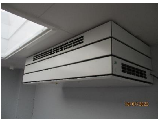
154. Airmaster ventilation unit. Library.
