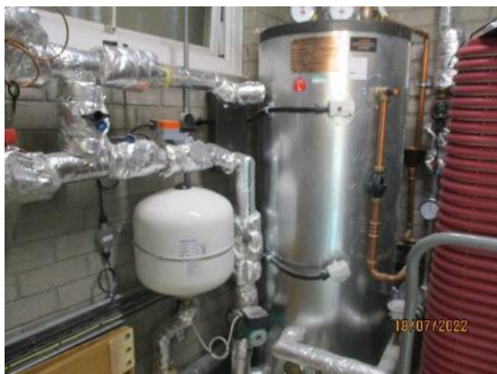
134. Calorifier 1 – hot water system storage hall cupboard.
