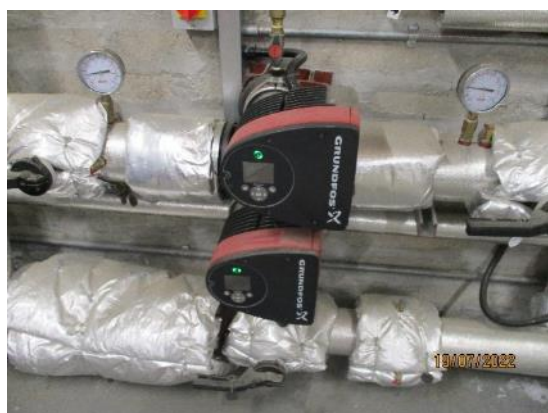
128. Pumps – main school heating. – Plant room
