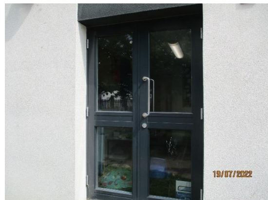
30. Fire exit double, glazed doors
