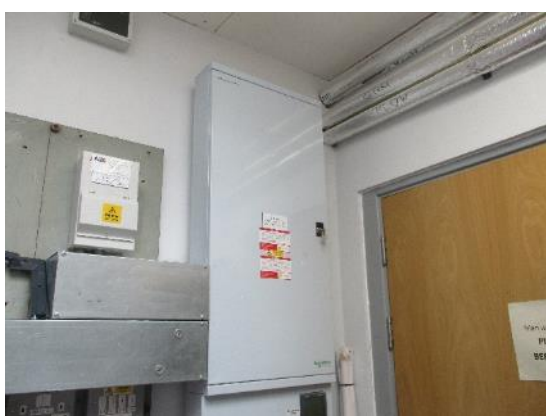
158. Electrical distribution board – switch room
