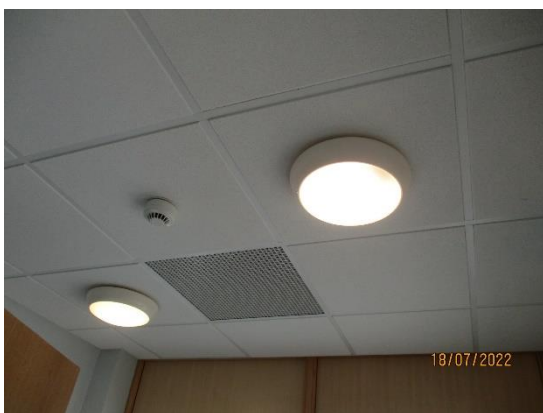
69. Suspended ceiling tiles
