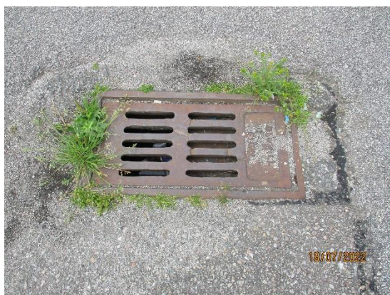
218. Partially blocked playground drainage
