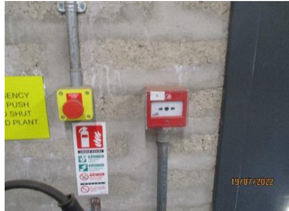
143. Gas safety stop push button – plant room.
