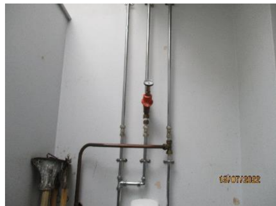
141. Pipework – cold water terminations at outlets.
