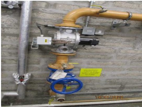
142. Gas pipework – main solenoid control valve. Plant room.
