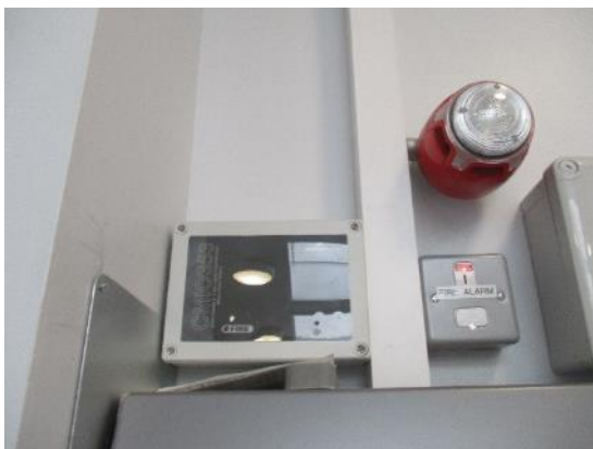
182. Fire alarm strobe and mag door disable interface.
