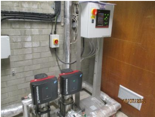
138. Cold water distribution – booster pump set.
