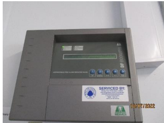
179. Fire alarm repeater panel. Main school.
