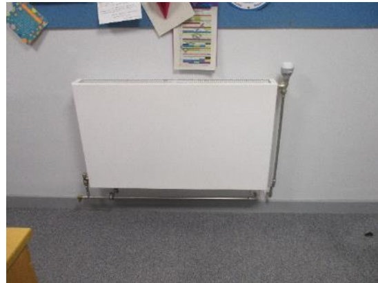
133. Radiator – typical. Deputy head office.
