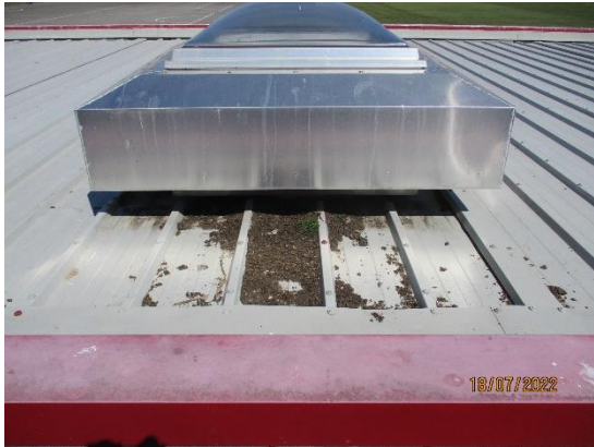
7. Roof cleaning required
