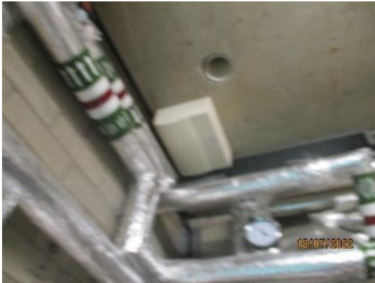
136. Pipework – hot water distribution.
