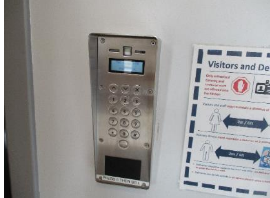
187. Paxton door entry control system camera and keypad.
