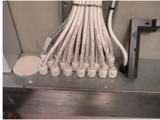
161. General wiring – switch room.
