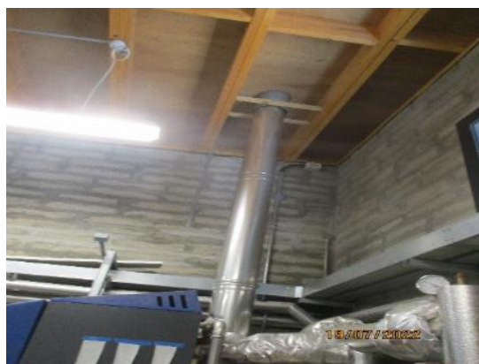
125. Gas boiler stainless steel flue. Plant room.
