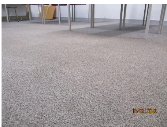
52. Ridges in concrete floor
