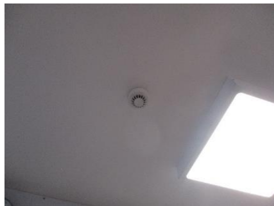
183. Fire detector head. HT office.
