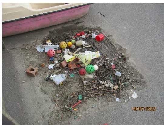
219. Partially blocked Nursery drainage
