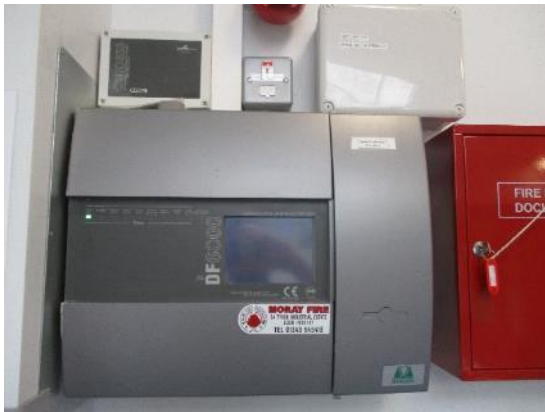
178. Fire alarm control panel. Main school.
