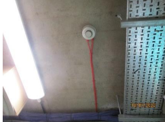
181. Fire alarm detector head and wiring. Main school.
