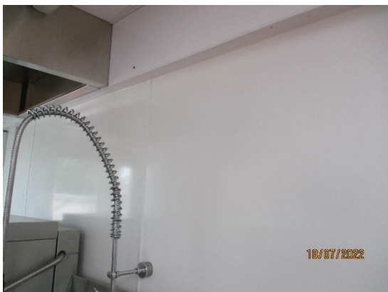
86. Wetwall in commercial kitchen
