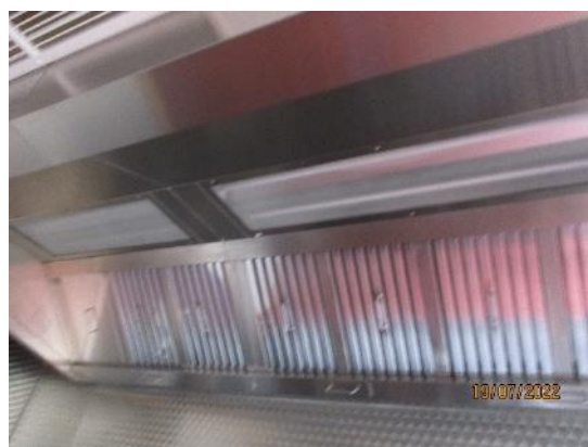
151. Extract fan and canopy. Main kitchen cooking appliances.
