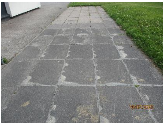
206. Cracked / damaged PCC slabs
