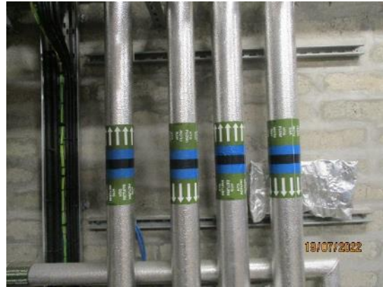
131. Pipework main heating system. Plant room.
