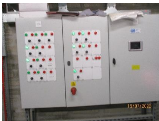
127. BMS heating control panel. Plant room.
