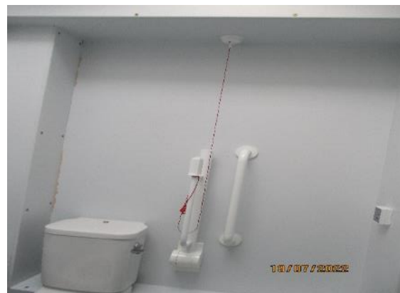
189. Disabled access alarm pull chord system.
