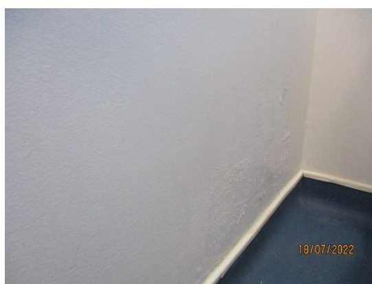
81. Damaged plasterboard surface
