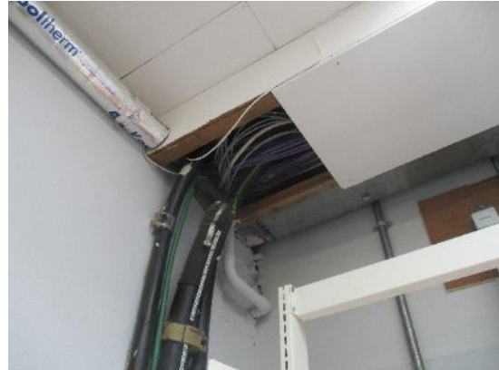
163. Sub mains supply cabling. Switch room.
