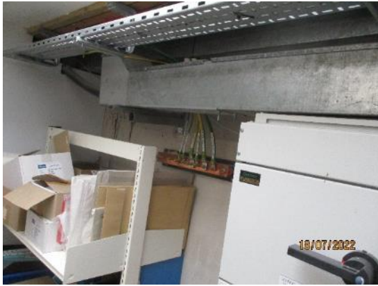
160. Main earth bar and isolator. Switch room.
