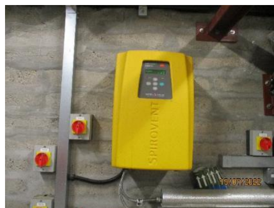
129. Degassing unit. Main heating system – Plant room.
