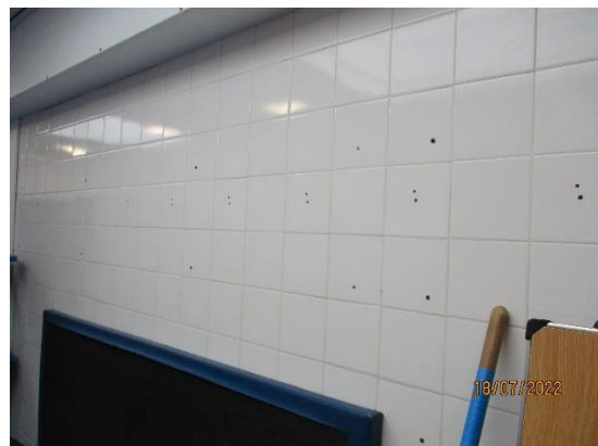
87. Damaged ceramic tiled walls
