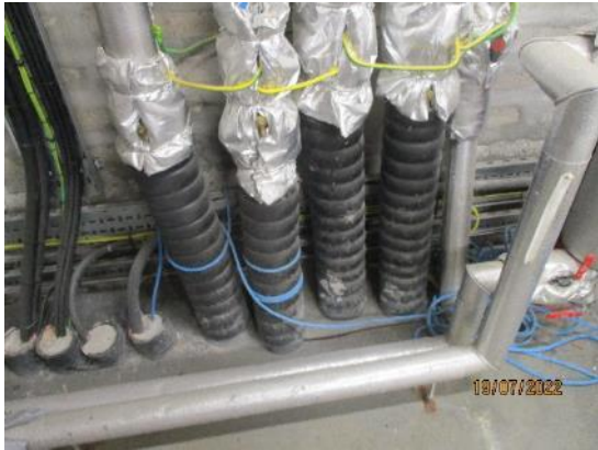
130. Pipework main heating system. Underground from plant room to main building.
