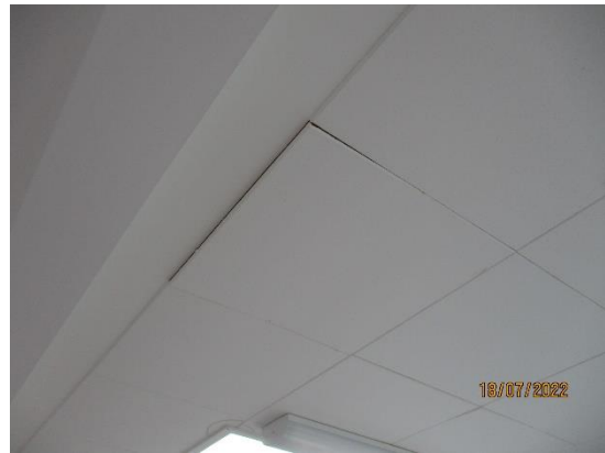
66. Loose fibre tiles
