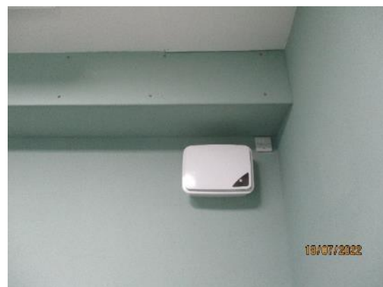
147. Extract fan – wall mounted typical.
