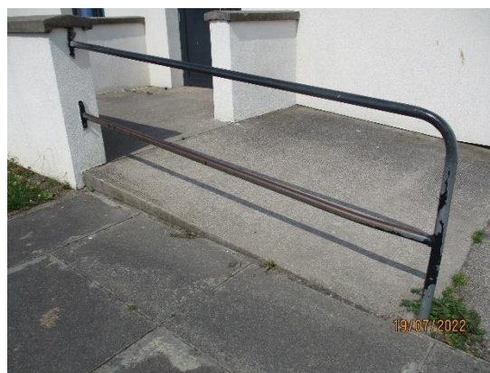
50. Tubular guard rail to fire exits
