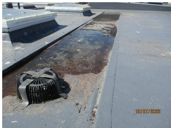
12. Flat roof gutters ponding
