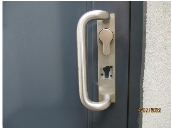
34. Damage to fire escape door ironmongery
