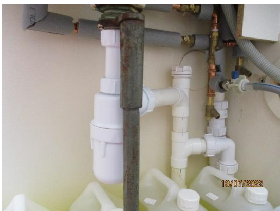
98. PVC waste pipes
