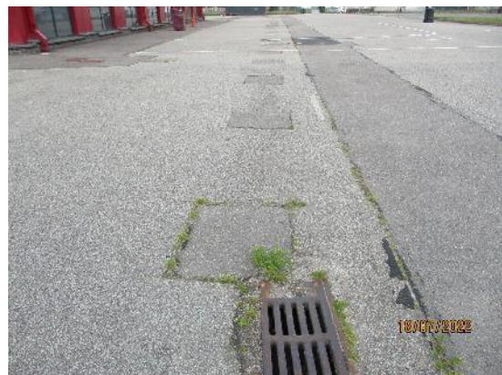
201. Cracked, patched playground
