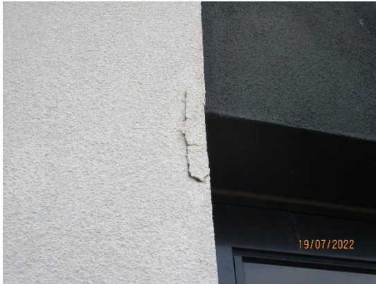
25. Damage to external insulation
