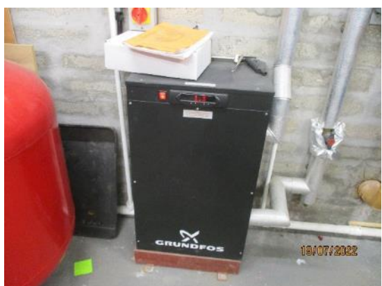
126. Pressurisation unit heating system – plant room.
