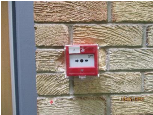
180. Fire alarm call point. Main school hall.- Typical.
