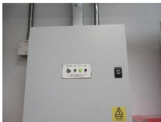
157. Hall ventilation units control panel.
