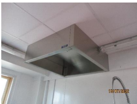
150. Extract fan and canopy. Main kitchen/dishwasher.
