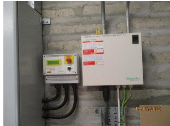
145. Gas safety system automatic control panel.
