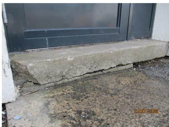
45. Broken concrete step to fire exit
