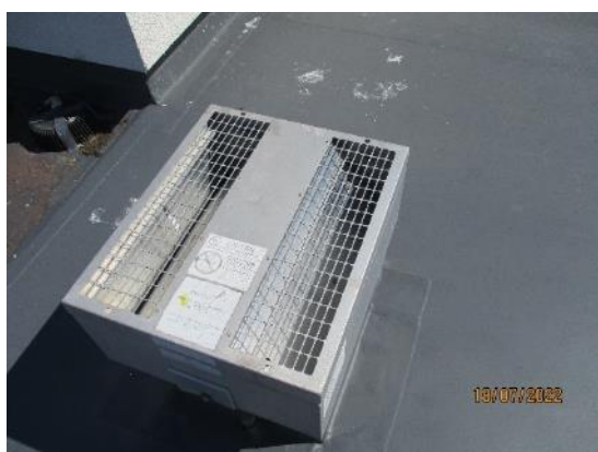
148. Extract fan – roof mounted. Kitchen roof.
