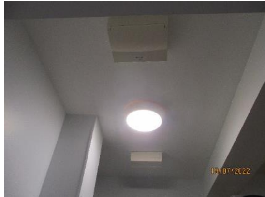
175. Lighting – main school store.
