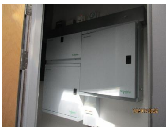
159. Electrical distribution boards – lighting and power
