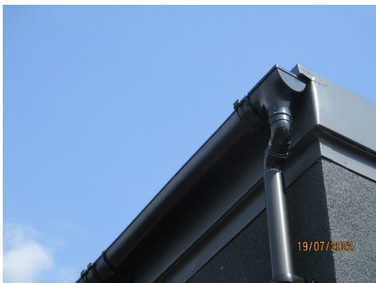
11. Gutter to boiler house
