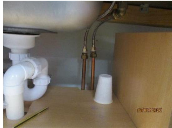
137. Pipework – hot water termination at outlets.
