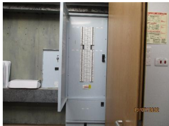
165. Electrical distribution board – main school typical.
