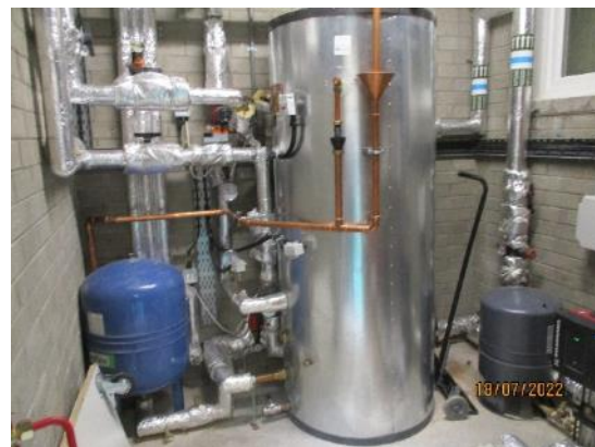
135. Calorifier no.2 hot water system. Hall cupboard.
