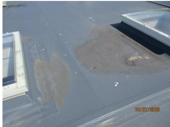
4. Areas of ponding
