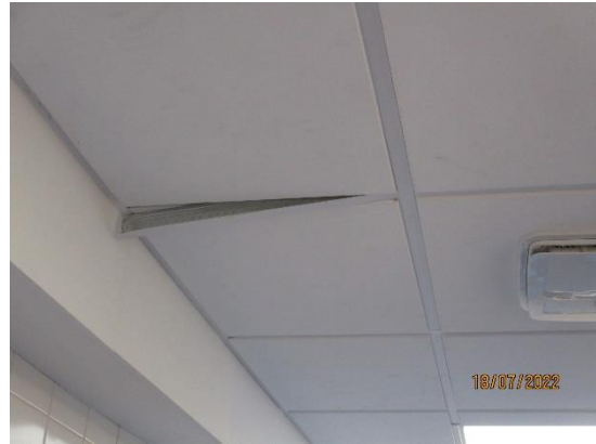
72. Damaged suspended ceiling tiles
