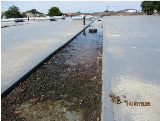
13. Partially blocked gutters
