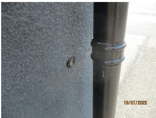
17. Boiler house downpipes – broken brackets
