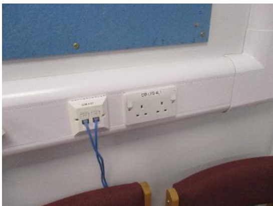
164. Electrical sockets/accessories. Typical.
