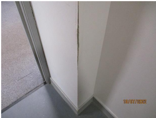
82. Damaged corner tape
