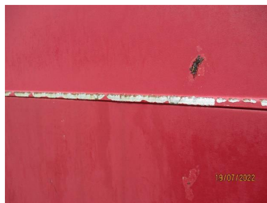
40. Peeling and flaking paint
