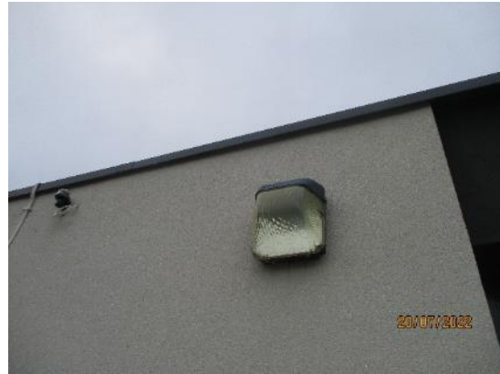
173. External lighting. Typical.
