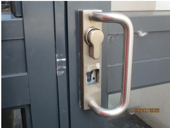
33. Damage to fire escape doors
