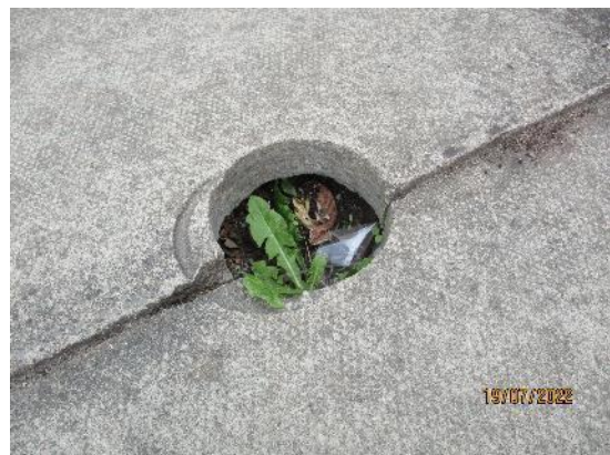
207. Holes in Nursery playground
