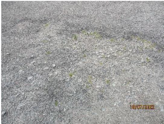
198. Eroded surface and potholes
