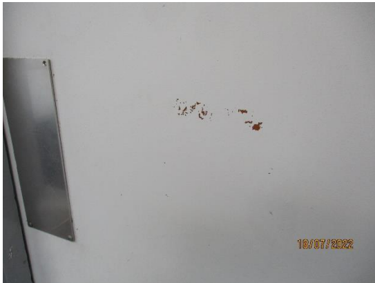
112. Chipped paint to timber doors
