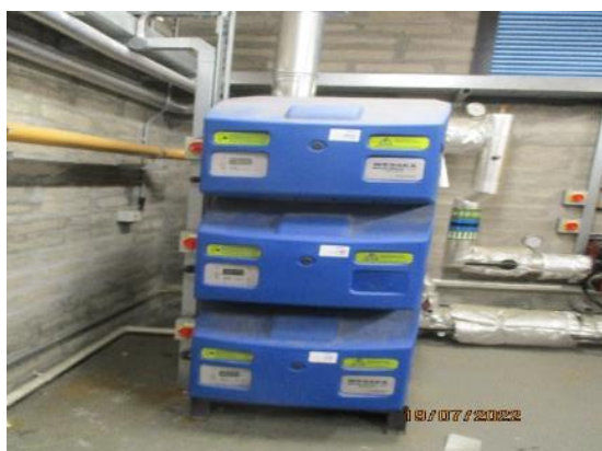
124. Natural gas modular boiler unit – 3 modules
