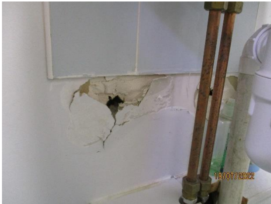
84. Damaged plasterboard walls
