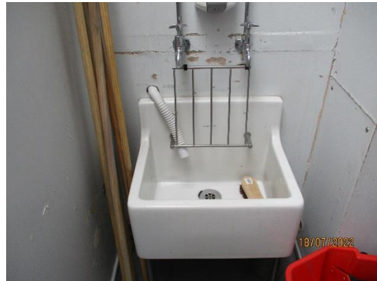
108. Butler cleaners sinks
