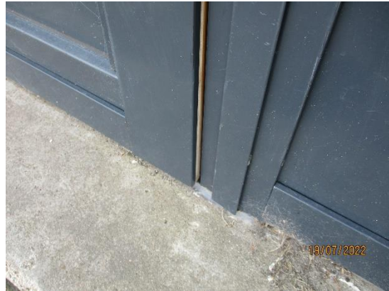
32. Poor fitting fire escape doors
