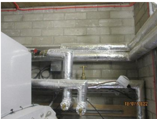
140. Pipework – cold water distribution at tank.
