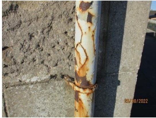
26. Cracked cast iron downpipes
