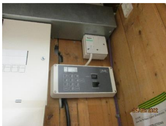
223. Period bell system. Digital control programmer.
