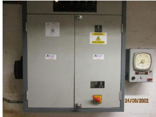
185. Heating system control panel. Boiler house.
