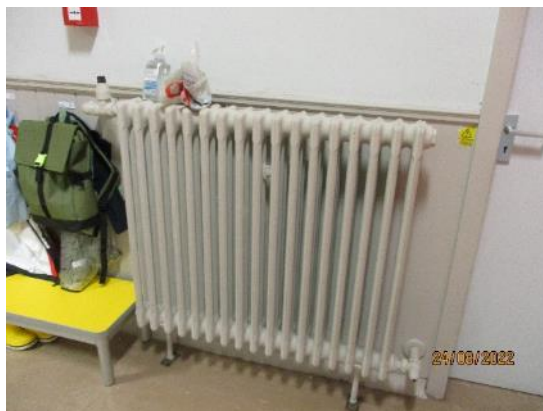
188. Cast iron radiator. Typical.
