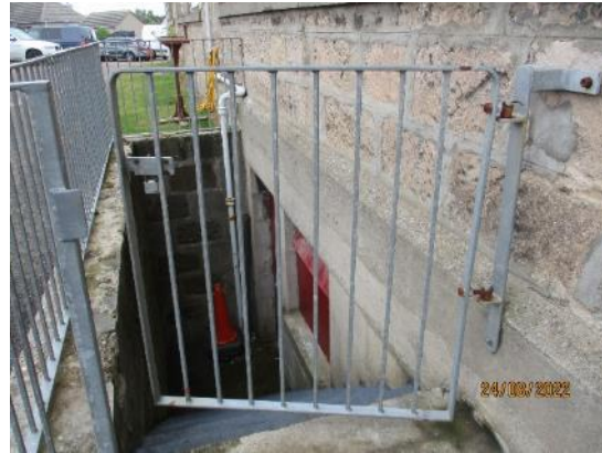
251. Galvanised gate to Boiler House
