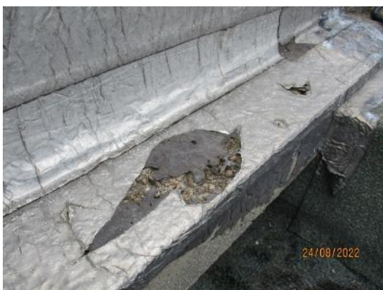
11. Perforated previous repairs
