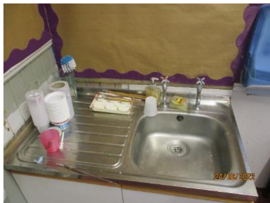
168. Typical sink with pillar taps
