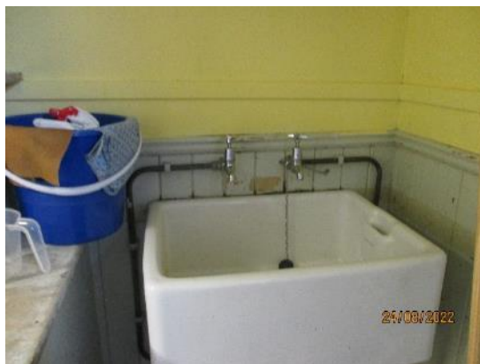
194. Pipework – hot water. Copper / cleaners room.
