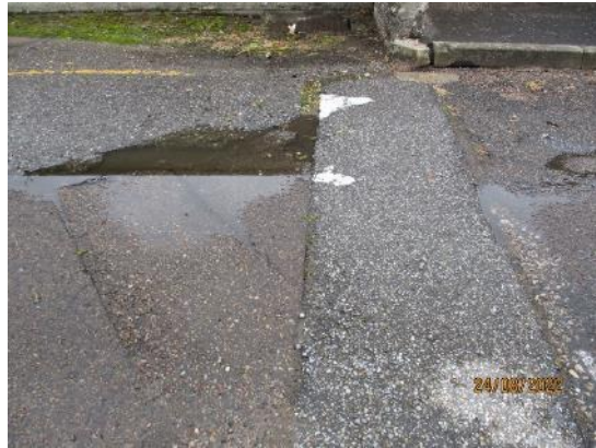
233. Potholes and ponding water
