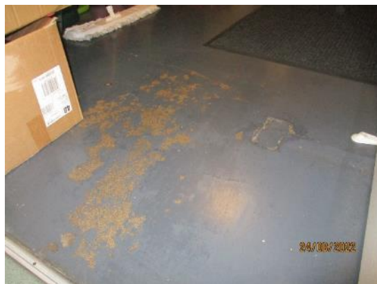
85. Uneven concrete floor
