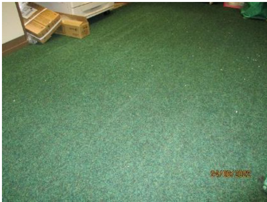
80. Wrinkled, loose carpet
