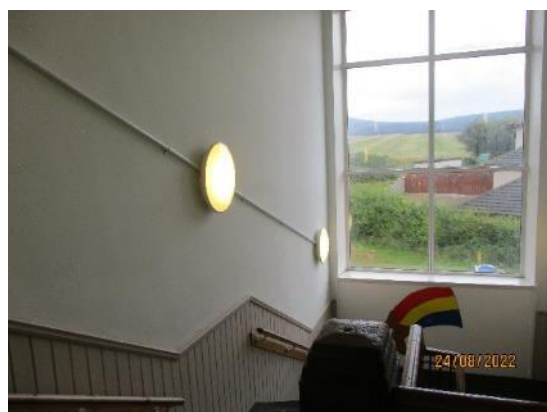
210. Lighting – stairs example.
