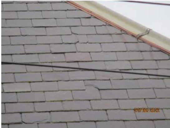
7. Isolated slipped and broken slates
