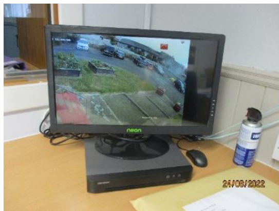
231. CCTV system processor and monitor. Reception office.
