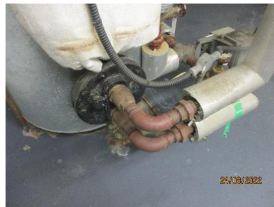
195. Pipework – hot water primary at calorifier.
