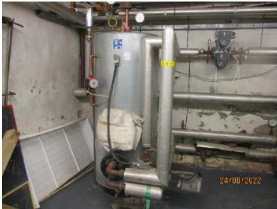
192. Hot water storage calorifier. Plant room.
