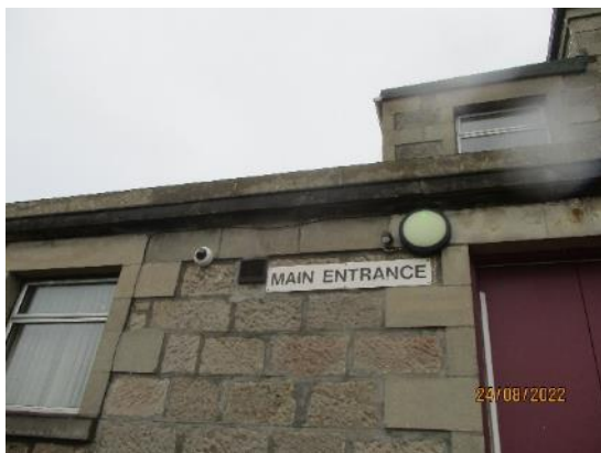
230. CCTV fixed external camera. Main entrance.
