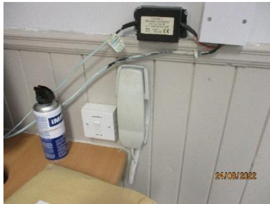
227. Security door control system. Handset.
