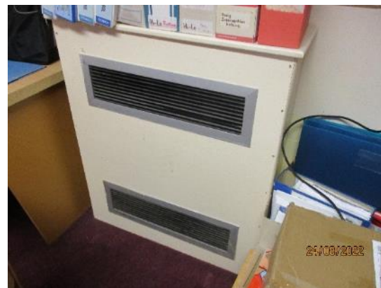
189. Convective heater – staff room.
