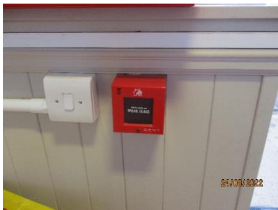
219. Fire alarm system device. – Call point.
