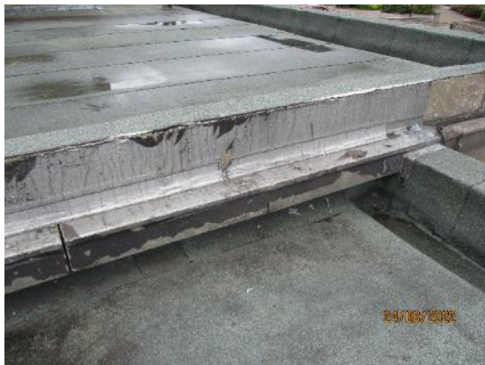
10. Previous poor quality repairs
