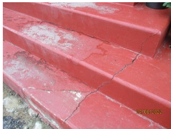
61. Cracked steps to front door
