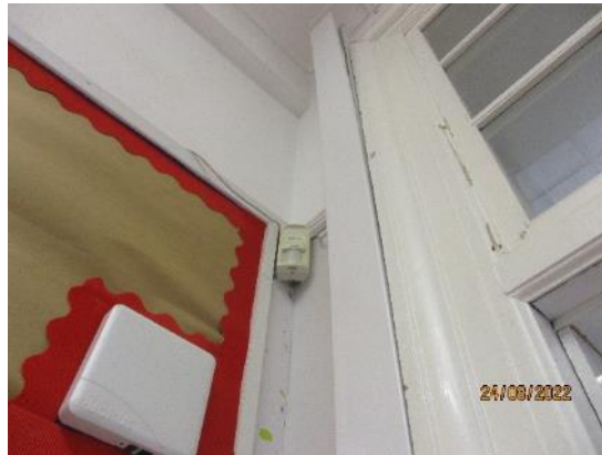
229. Intruder alarm system – PIR example.
