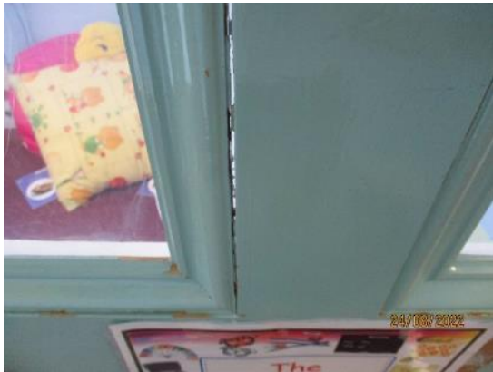
135. Gaps to glazed panels
