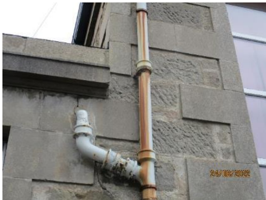
21. Corroded cast iron downpipes
