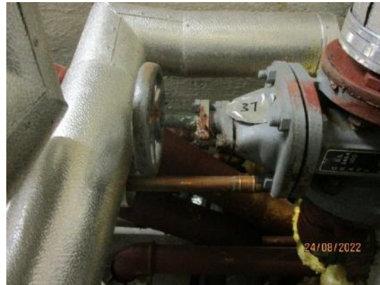
187. Heating system pipework and valves. Boiler house.
