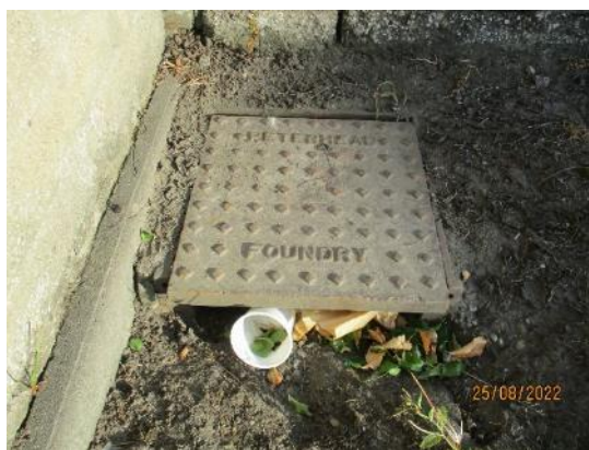
258. Partially blocked drainage
