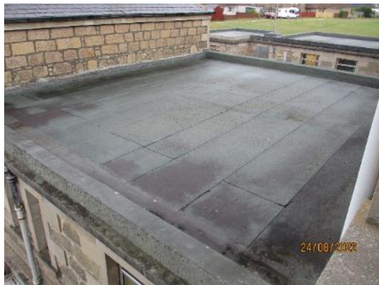
9. Silt on felt roofs
