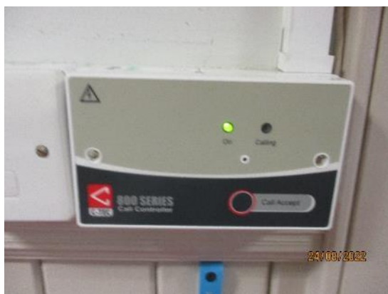
224. Disabled toilet alarm system – alert panel.
