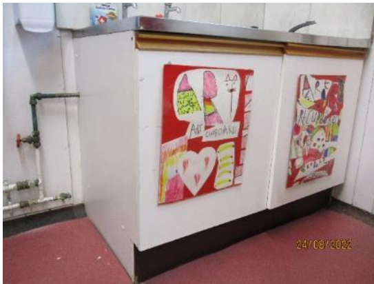
163. Base units in poor condition
