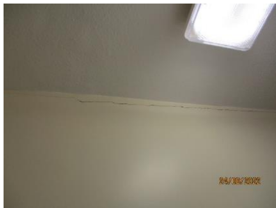
114. Failing taped joints
