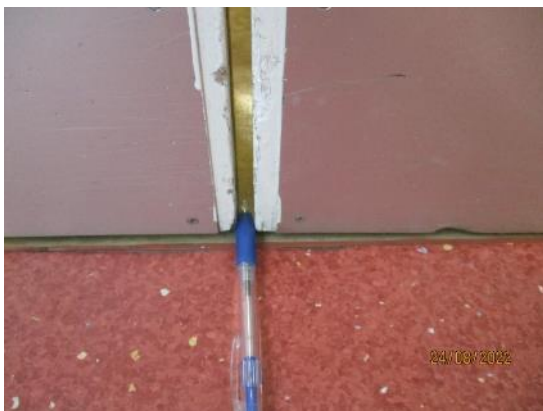
131. Large gaps between fire doors
