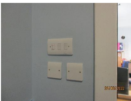
213. Lighting – control switch example. Typical.
