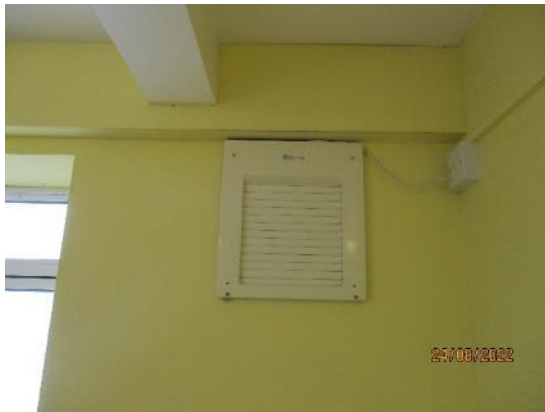
202. Extract fan. Boys toilets.
