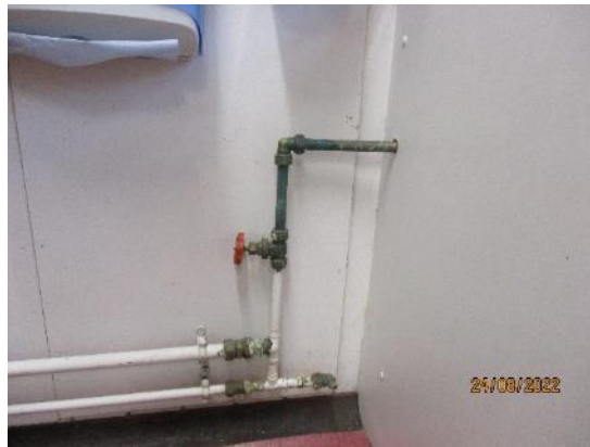
197. Pipework – cold water distribution.
