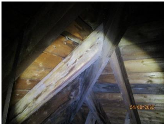
3. Evidence of previous water penetration
