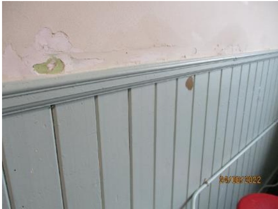
115. Spalling plaster walls
