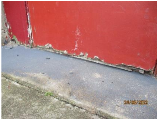
37. Rot in bottom of timber doors
