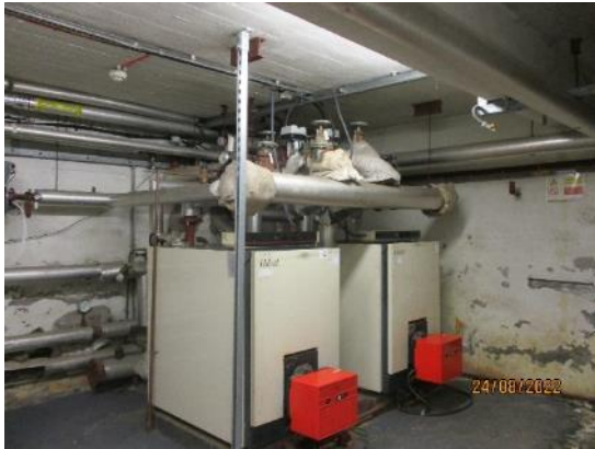
184. Gas boilers – boiler house.
