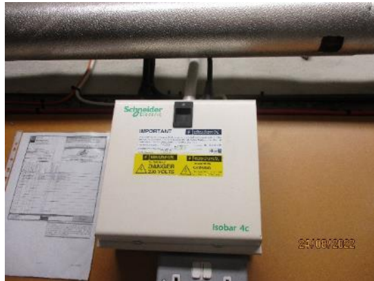
205. Distribution board. Power – boiler house.
