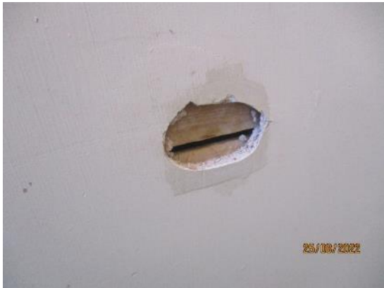
117. Damage to lath & plaster walls
