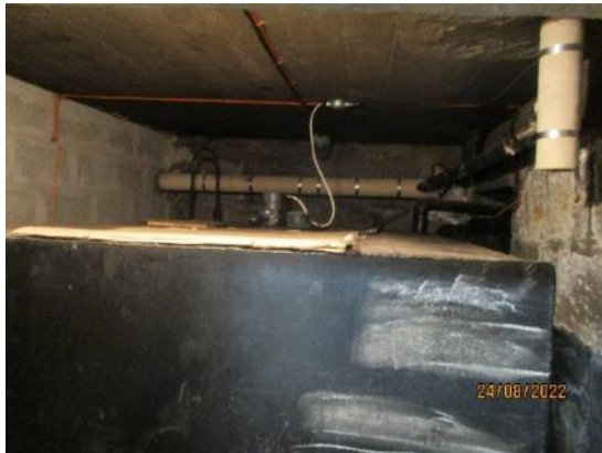
198. Oil storage tank. Basement 0/36
