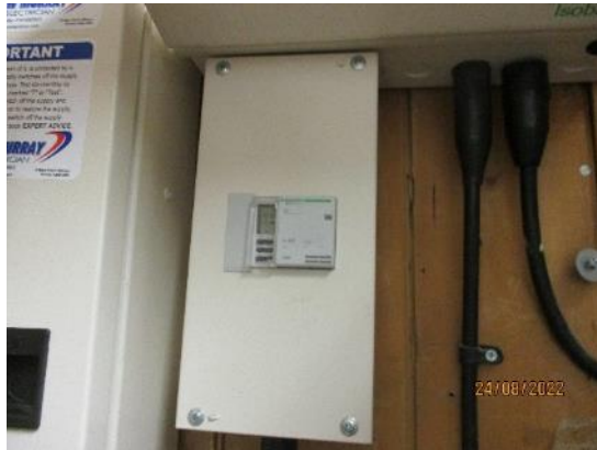
217. External lighting digital programmer – control.
