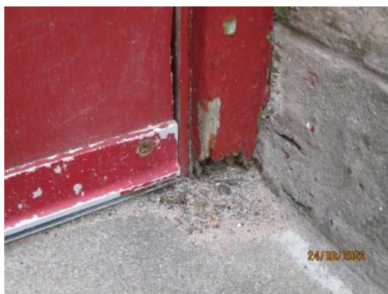
35. Wet rot in timber frame
