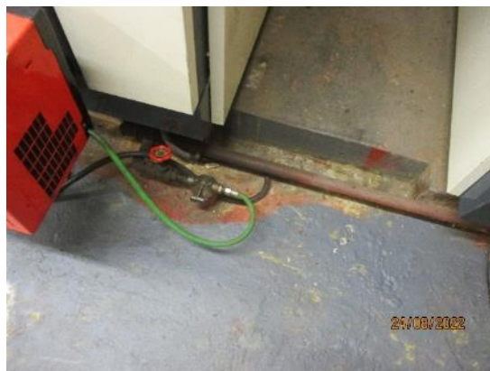
201. Oil supply pipework at boilers.
