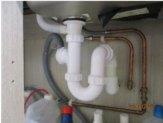
171. UPVC waste pipes
