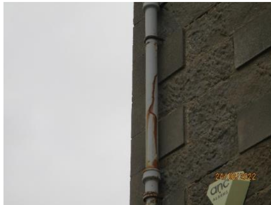
20. Cracked cast iron downpipes
