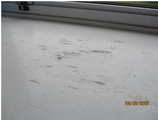
127. Timber window sills
