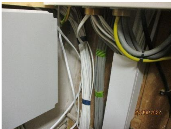
206. General wiring. Print room cupboard.
