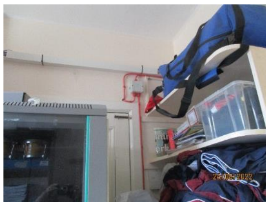
221. Fire alarm system wiring – store cupboard.
