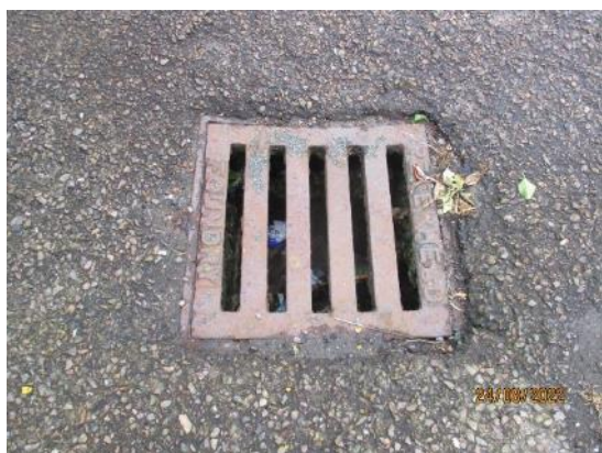
257. Surface water drainage
