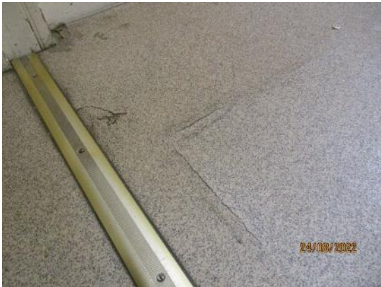
76. Damaged sheet vinyl
