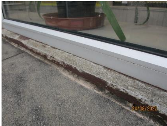
55. Timber window sills
