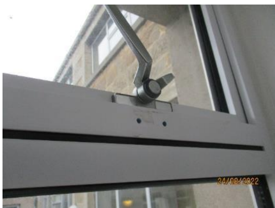
53. Lever handles and missing keepers
