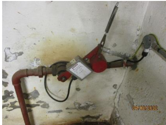
199. Oil pipework / safety shut off valve.
