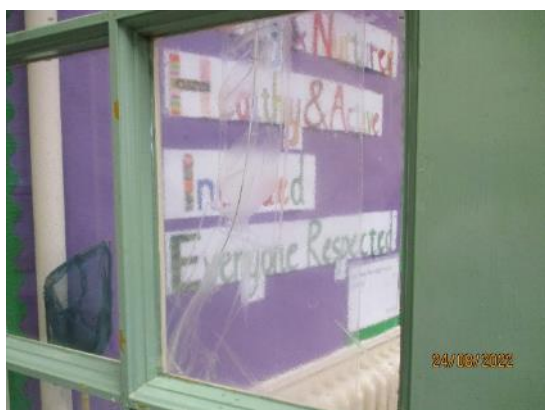
141. Broken glass in doors
