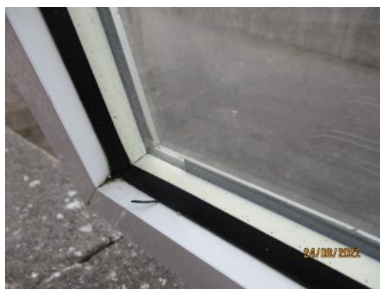
46. Double glazing – missing seals
