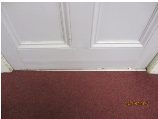
137. Doors twisted within frames
