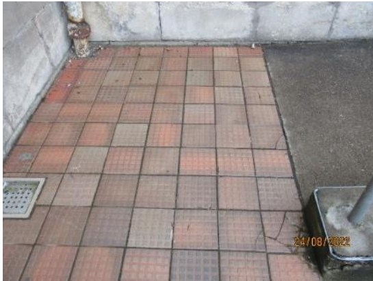
68. Quarry tiles loose and broken
