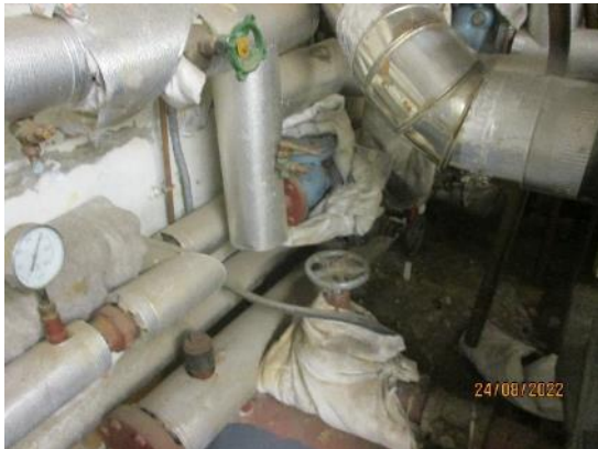
186. Heating system pipework. Boiler house.
