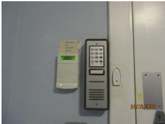
226. Security door control intercom unit.
