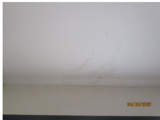
102. Damaged lath & plaster ceilings
