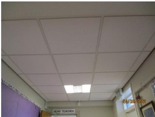
99. Suspended ceiling tiles
