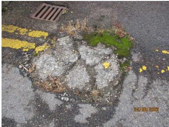
234. Surface patched and breaking up
