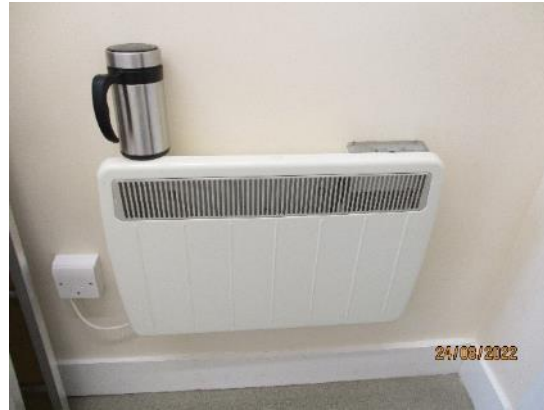
191. Electric convector heater. Access WC
