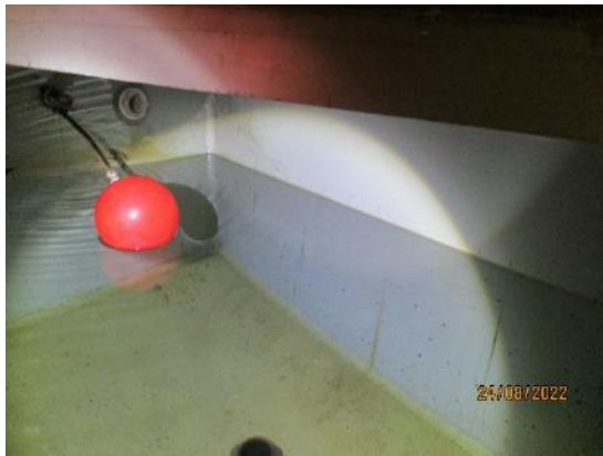
196. Cold water storage tank. Attic space.
