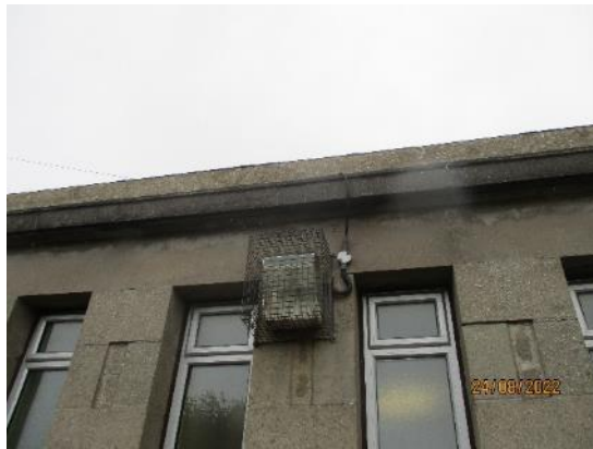
215. External lighting typical.
