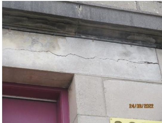
28. Cracked lintol above main entrance
