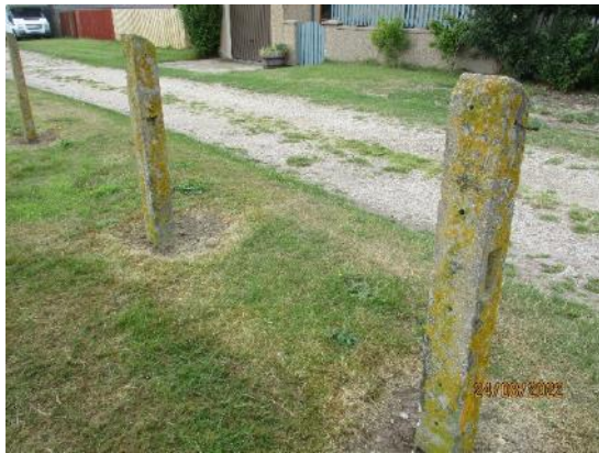
244. Missing wire fence
