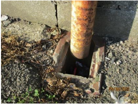
25. Back inlet gullies with missing gratings
