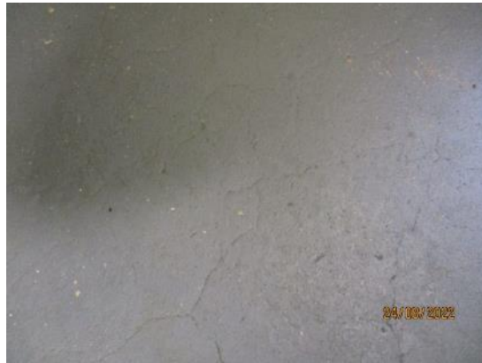
83. Crazed concrete floor
