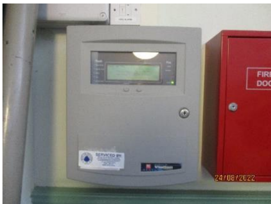
218. Fire alarm system control panel.
