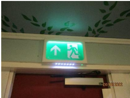
214. Emergency lighting. Typical.
