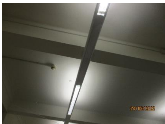
208. Lighting. Classroom typical.
