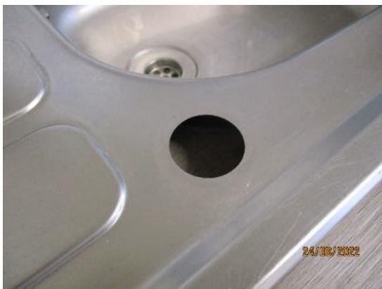
167. Broken blanking plates
