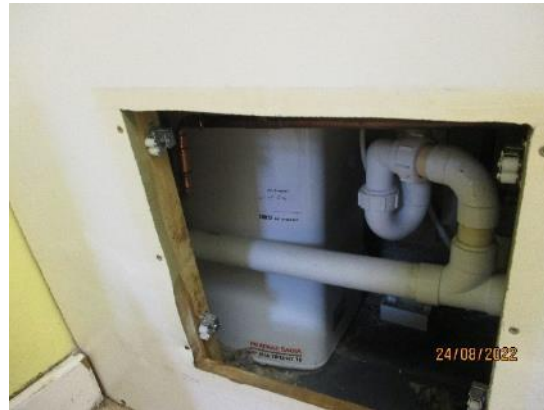
193. Hot water point of use heater. Girls toilets.
