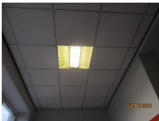
209. Lighting – corridor typical.
