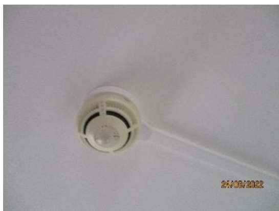
220. Fire alarm system device. Detector head.
