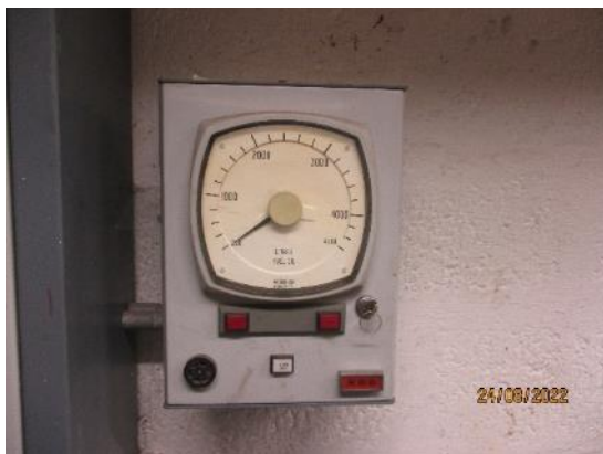
200. Oil tank – over fill alarm system unit.
