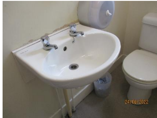
154. Wall hung basins (staff)
