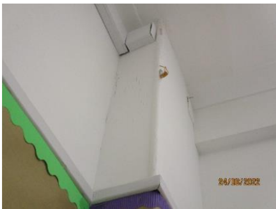
113. Damage to lath & plaster walls
