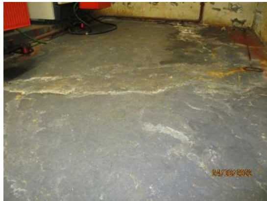
87. Uneven boiler house concrete floor
