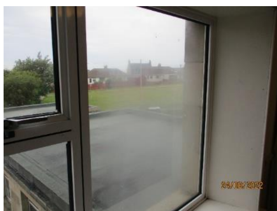
48. Fogged double glazing
