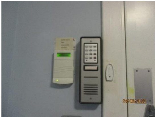
228. Intruder alarm system control panel.
