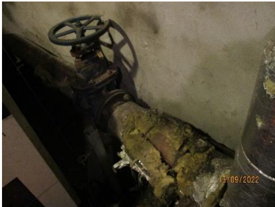
206. Pipework – heating system. Plant room 0/1
