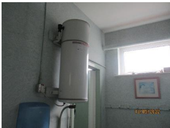
214. Hot water storage cylinder – Girls toilets.
