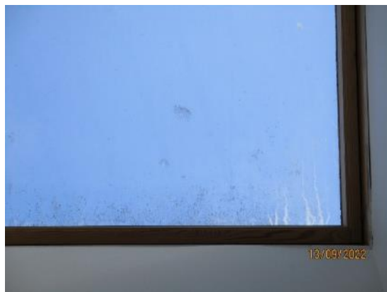
78. Failing solar film
