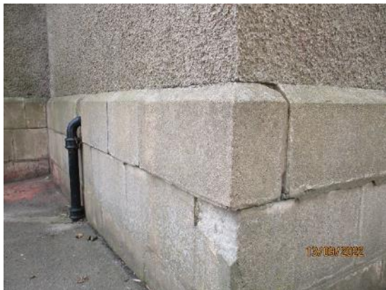
52. Slipped masonry above DPC
