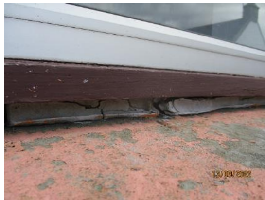
72. Failed sealant below window sills
