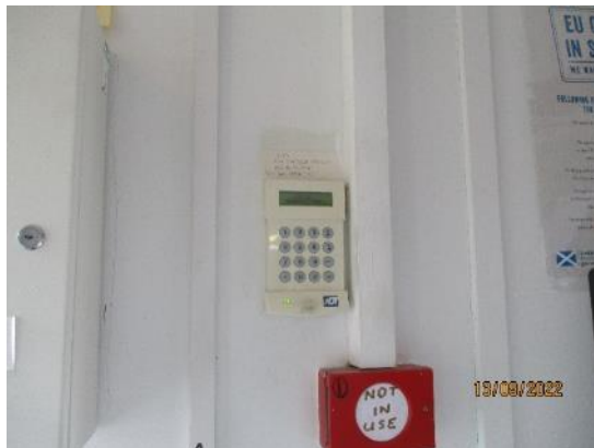
242. Intruder alarm keypad – entrance lobby.
