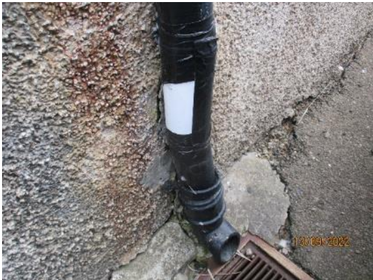
39. Impact damaged cast iron
