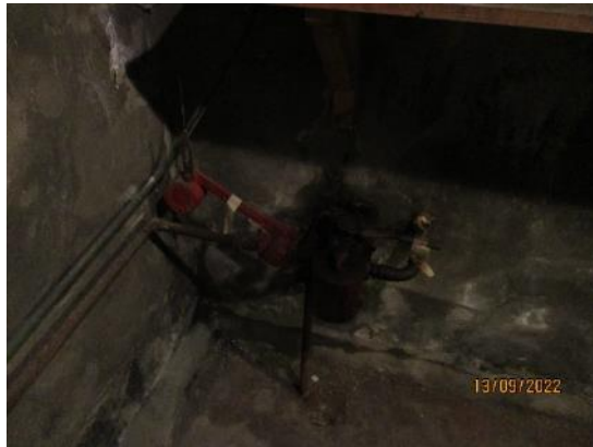
219. Oil supply auto shut off valve and pipework. 0/1
