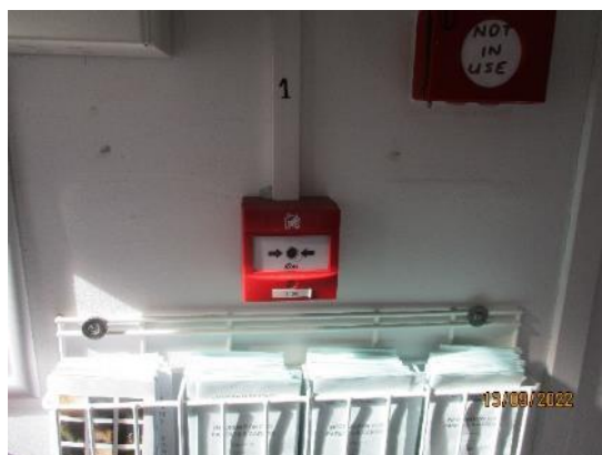
239. Fire alarm system call point. Typical.
