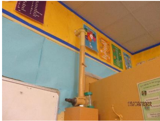
207. Pipework – heating distribution. Typical.
