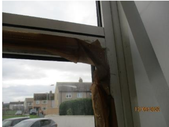
74. Windows taped where seals have failed
