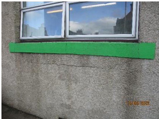
51. Cracking to external walls
