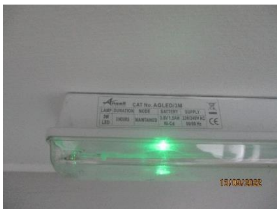
234. Emergency lighting – typical.
