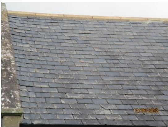
11. Slipped and broken slates
