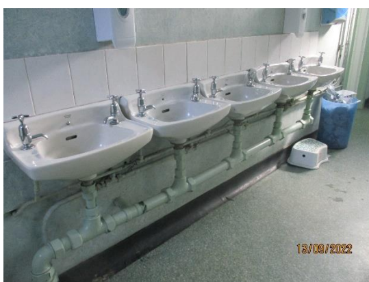
174. Basins in Girls Toilet
