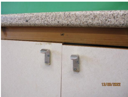
202. Missing handles, damaged base units
