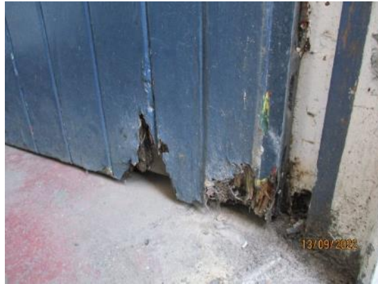
68. Rot at bottom of door
