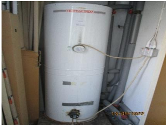
212. Hot water storage cylinder. Kitchen cupboard
