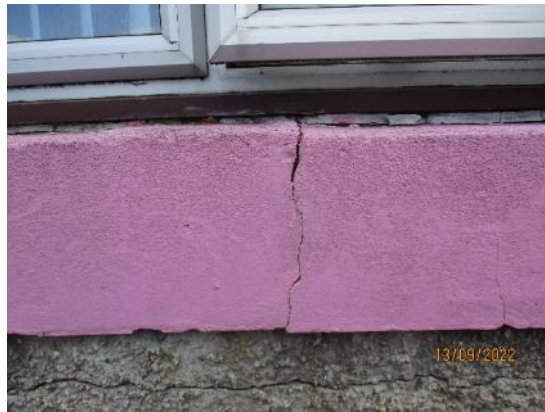
50. Cracked concrete window sills
