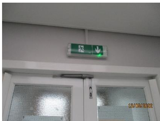
235. Emergency exit sign lighting. Typical.
