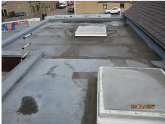
19. GRP roof, soiled
