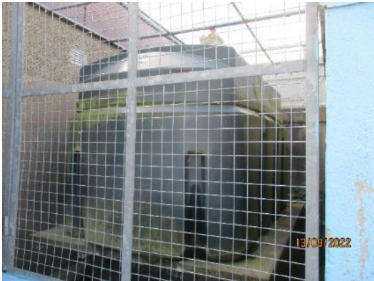
218. Oil storage tank in external bunded secure store.
