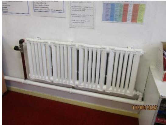
211. Radiator – cast iron section classroom
