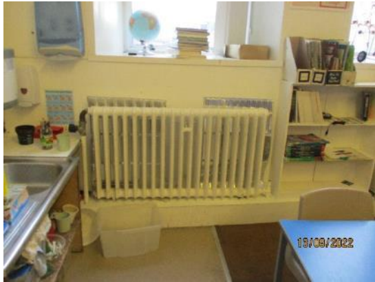
210. Radiator – cast iron column. Classroom
