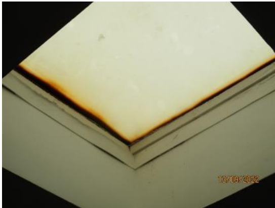
27. UV degradation of domed rooflights
