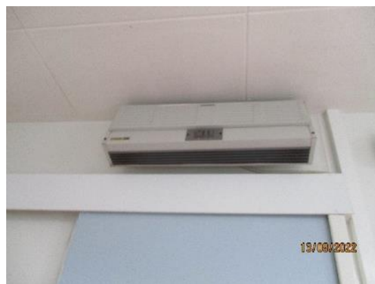
209. Electric fan heater - kitchen
