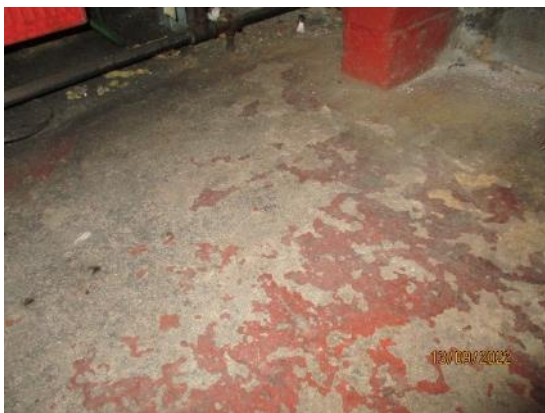
113. Worn concrete floors – Boiler House
