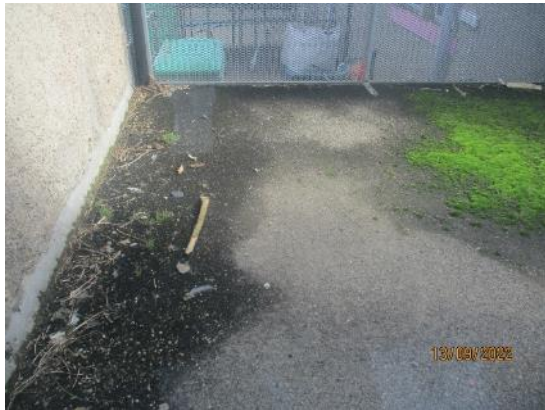
21. Felt roof – debris and vegetation
