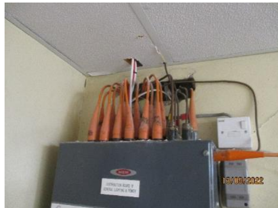
225. Distribution board and supply general wiring.
