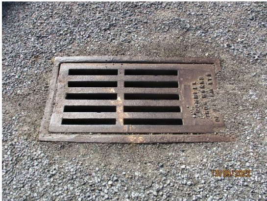
284. Playground road gully
