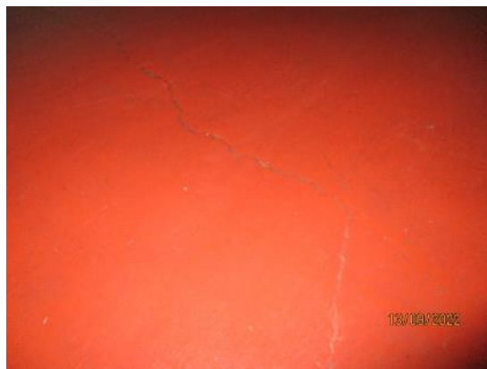
114. Cracked concrete floor – Boys Toilet
