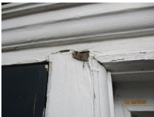
62. Rot in timber door frames
