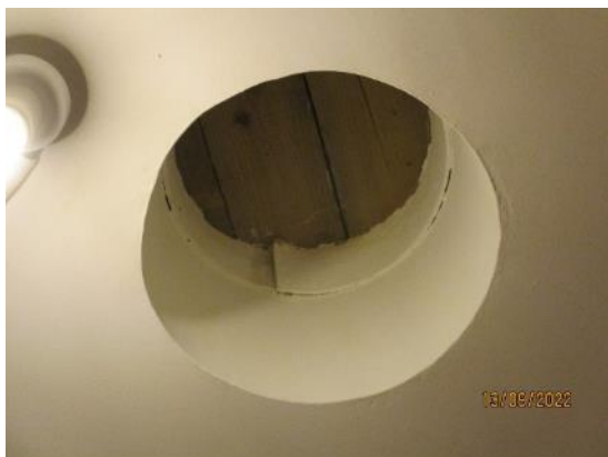
125. Redundant vent in Staff Toilet ceiling
