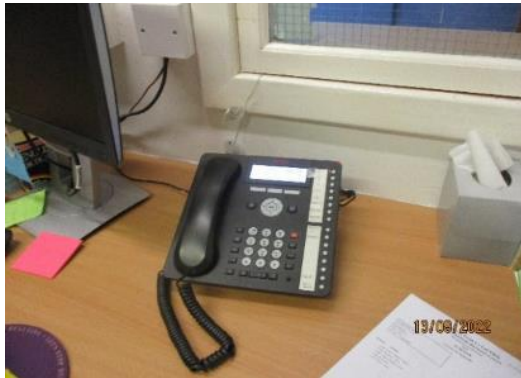
248. Phone system – reception office.
