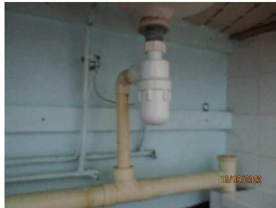
176. PVC waste pipes
