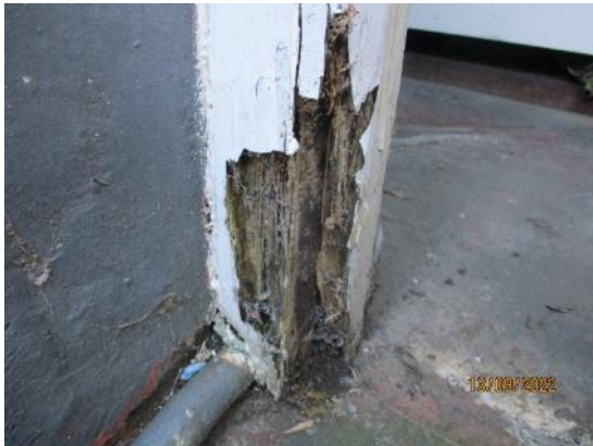
69. Rot in door frame
