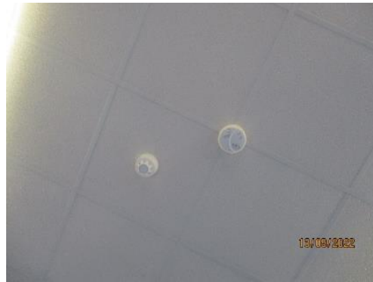
241. Fire alarm system detector head. Classroom.
