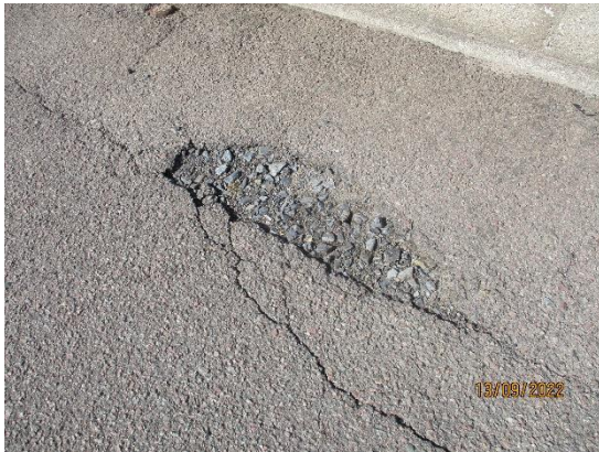
254. Surface erosion and potholes
