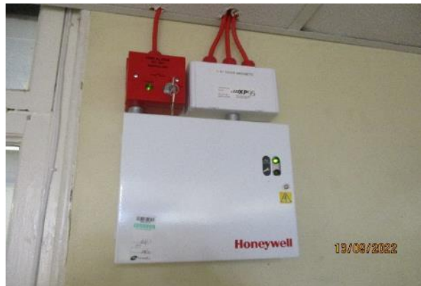
249. Entrance door magnet – control panel.
