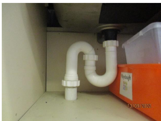
189. PVC waste pipes
