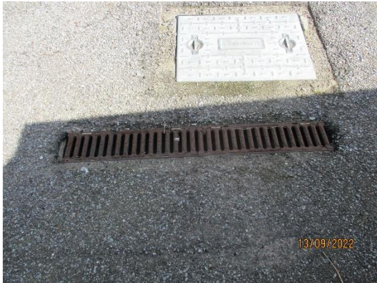
282. Car park channel drain
