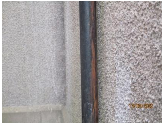
38. Cracked, corroded downpipes
