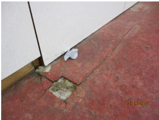
105. Damaged linoleum flooring
