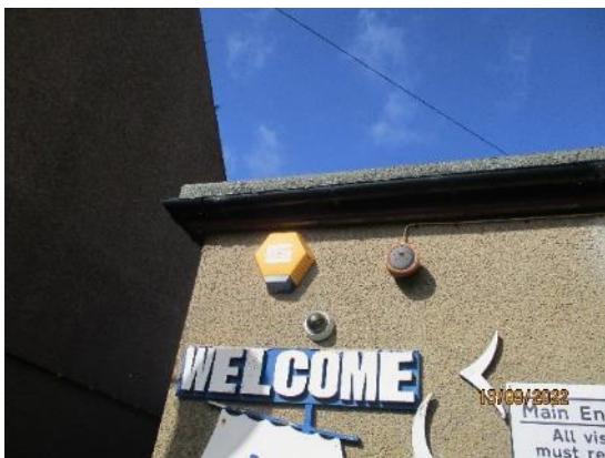
250. External CCTV camera.
