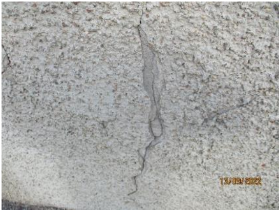
57. Cracked, spalling roughcast finish
