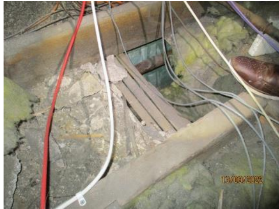
32. Missing insulation, damaged lath & plaster
