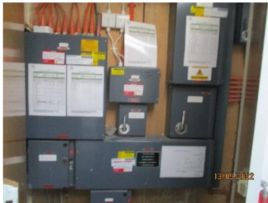
224. Switchgear and distribution boards.
