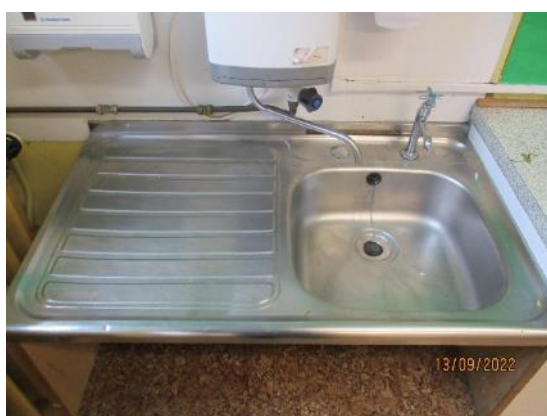
185. Stainless steel classroom sinks
