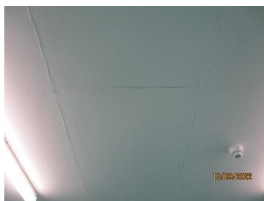
119. Plasterboard ceilings – failed taped joints
