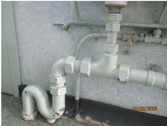
177. Copper waste pipes (Girls Toilet)
