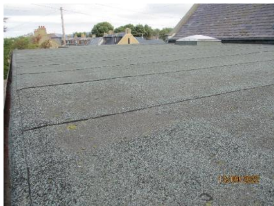
24. Surface erosion of felt roofs
