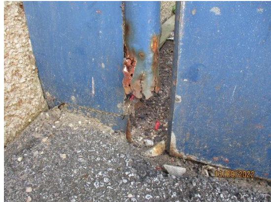
271. Corroded, broken post
