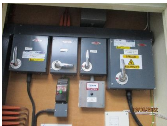
227. Fused isolators. Switchgear.
