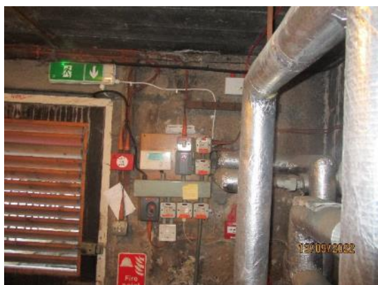
208. Heating controls – plant room 0/1
