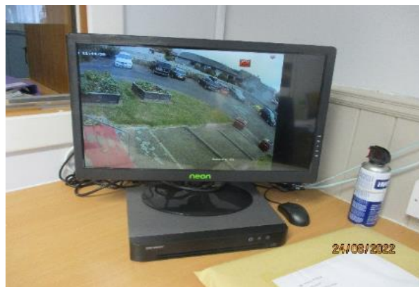
251. CCTV monitor and processor.
