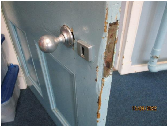
157. Wear and damage to classroom doors
