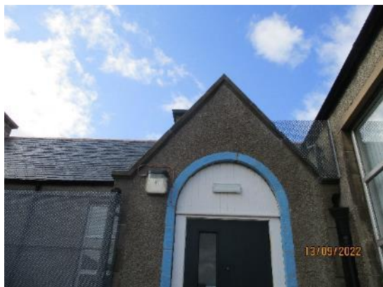
236. External lighting – typical.
