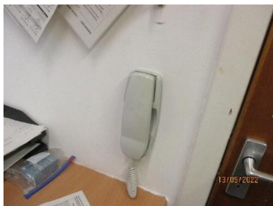
245. Security door access handset – reception office.
