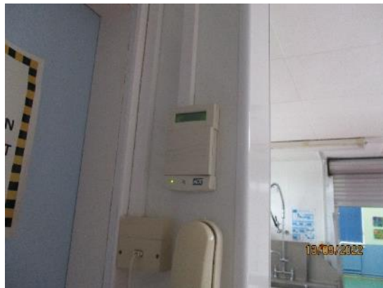
243. Intruder alarm keypad 2 – kitchen.
