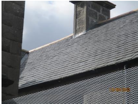
9. Irregular roof surface
