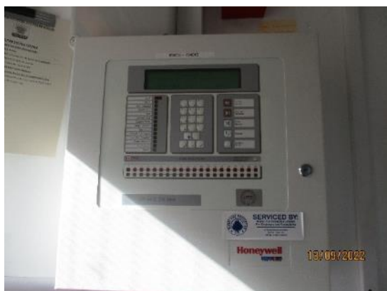
238. Fire alarm system control panel. Entrance lobby.
