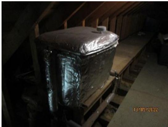
216. Cold water storage tank. Above dining hall.
