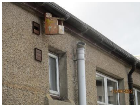
42. Damaged UPVC SVP's
