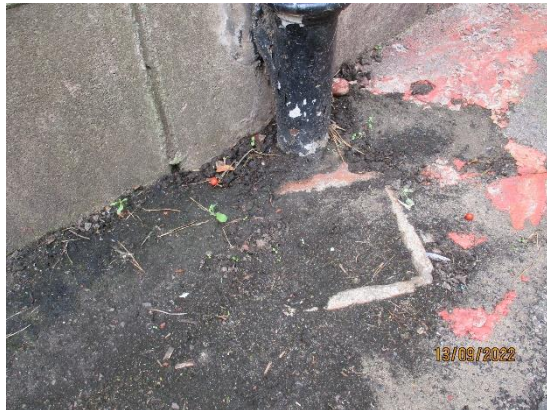
285. Gullies at downpipes, blocked
