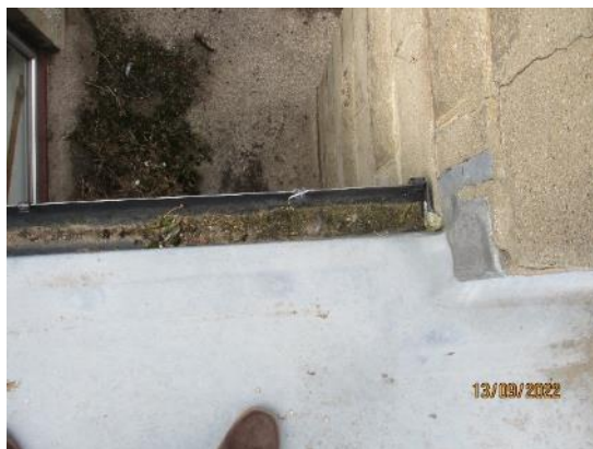
35. Some gutters require cleaning
