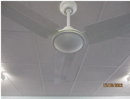
222. De stratification fan - classroom
