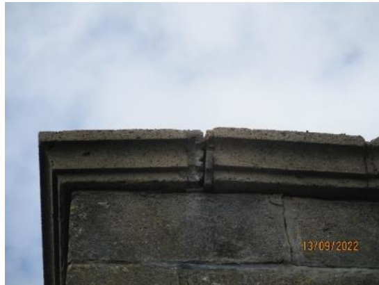
46. Missing pointing to copes
