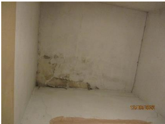
128. Damaged lath & plaster ceilings
