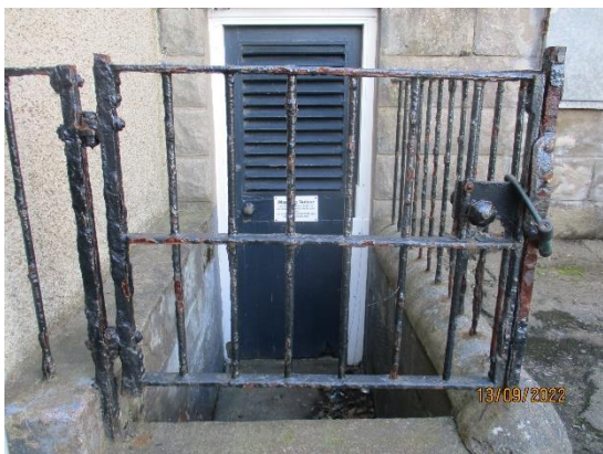
274. Metal railing gate with extensive corrosion
