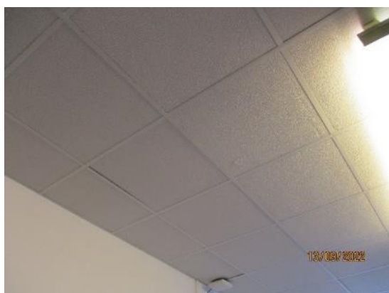
116. Suspended ceiling tiles
