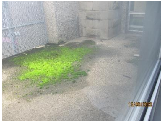
22. Moss on felt roof
