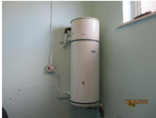
213. Hot water storage cylinder. Cleaners/boys toilets.
