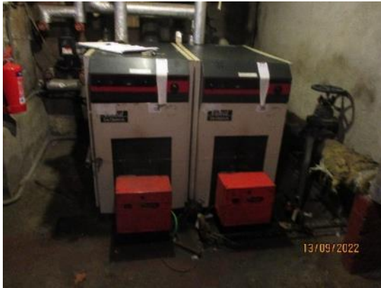
204. Oil fired boilers. Plant room 0/1
