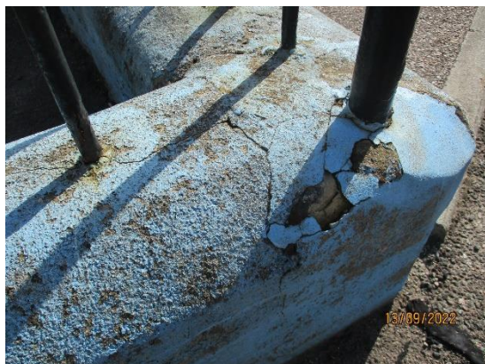
275. Coping to low level wall - cracked
