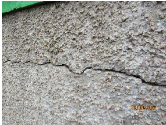
55. Cracking of roughcast finish
