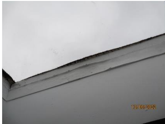
28. Distorted seals to rooflights
