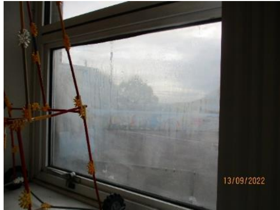
80. Fogged double glazing units
