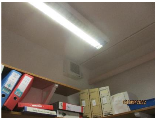
220. Extract fan – reception office.
