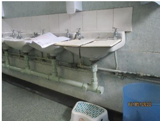
217. Pipework – cold water. Girls toilets.
