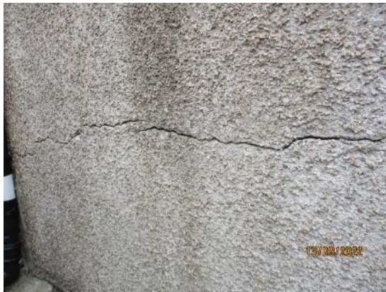
49. Cracking to external walls
