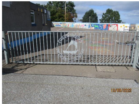
267. Galvanised vehicle gate to playground
