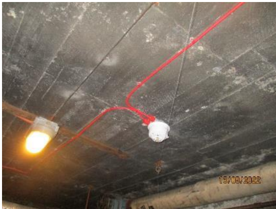
240. Fire alarm system wiring and detector head. 0/1
