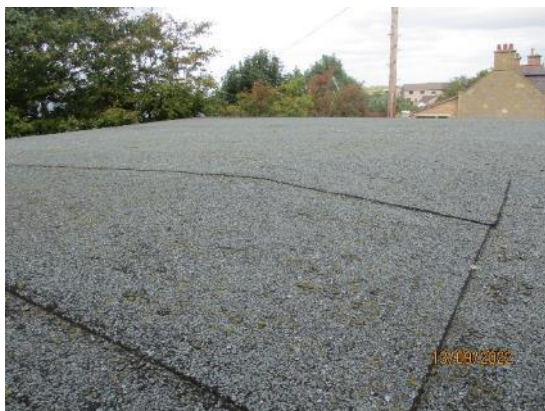
23. Falls on felt roof
