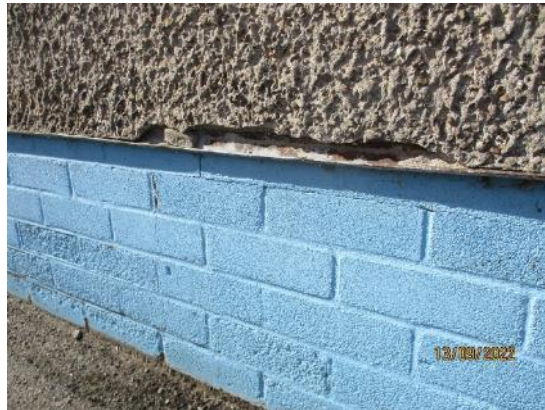
58. Missing roughcast at bellcast bead
