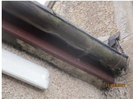
34. Cast iron gutters
