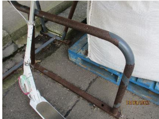
289. Corroded metal frame
