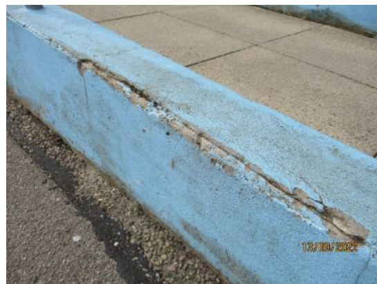
96. Damaged kerb wall
