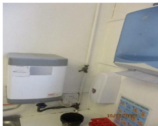
215. Point of use hot water heater. Typical.
