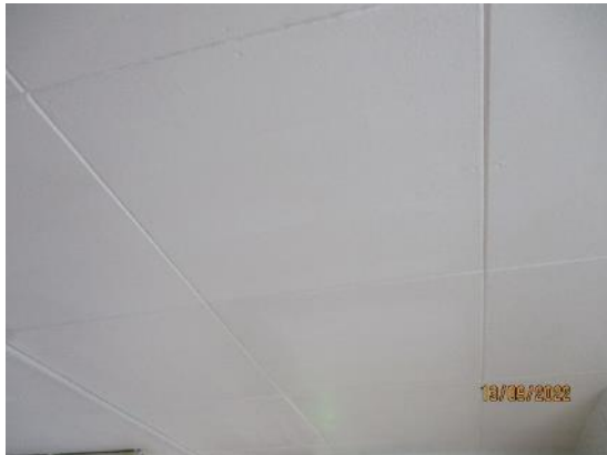
123. Ceiling tiles - Kitchen
