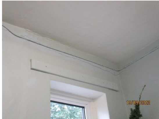
133. Cracks at high level
