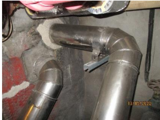
205. Boiler flues into brick chimney. Plant room 0/1
