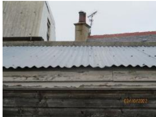
16. Uneven roof surface, no rainwater goods
