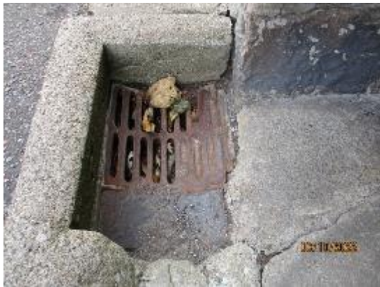
278. Part blocked road gully
