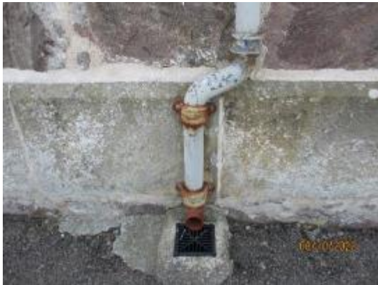
33. Downpipes to surface gullies
