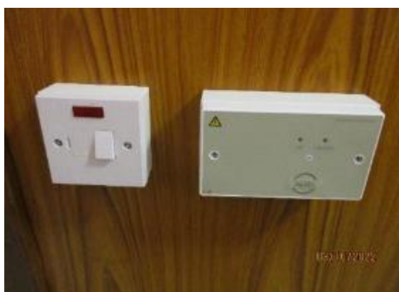
218. Disabled toilet alarm system panel. 1/12
