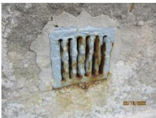
51. Corroded sub-floor vents
