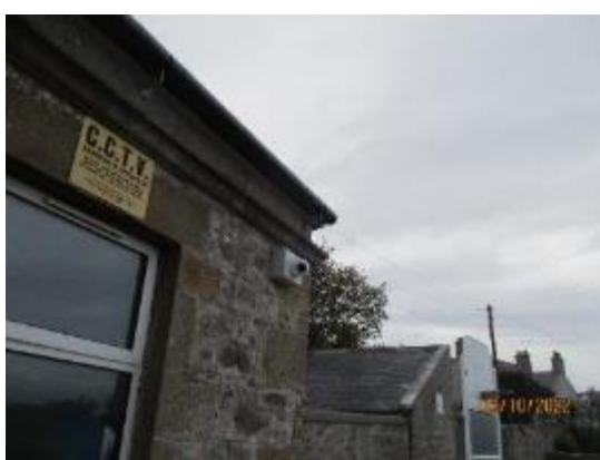
223. External CCTV camera. Main entrance.
