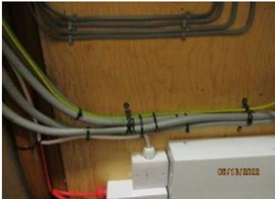
202. Sub mains cabling cupboard 1/22
