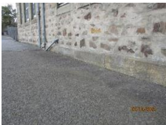
49. Ground level high in SW corner
