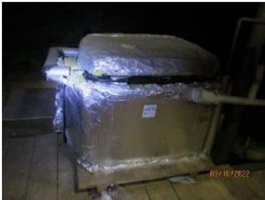
190. Cold water storage tank above 1/11 corridor.
