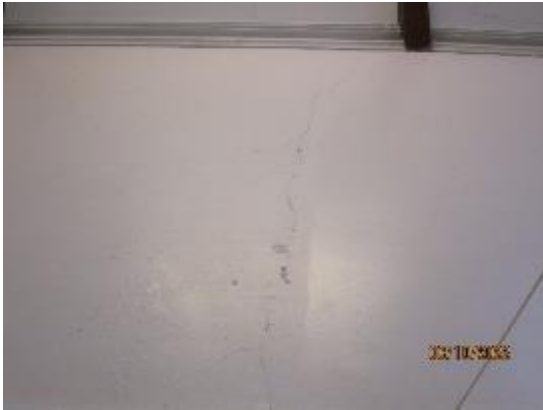
107. Lath & plaster walls cracked
