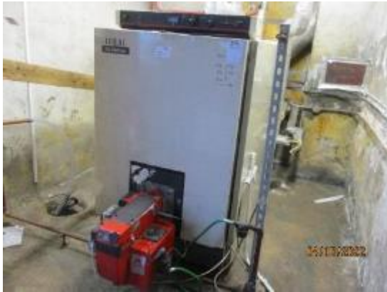
176. Boiler and burner. – Oil fired. Plant room 0/26
