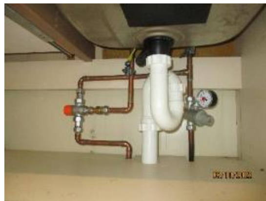
163. PVC waste pipes
