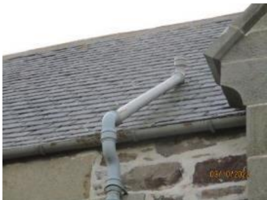
36. Cast iron soil vent pipes
