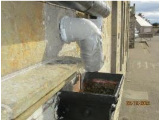
31. Damaged rainwater outlets
