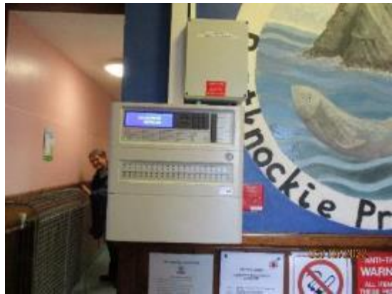
213. Fire alarm control panel. 1/1
