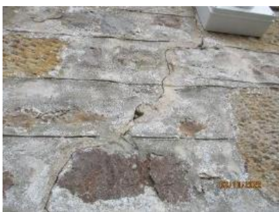
53. Pointing required to isolated cracking
