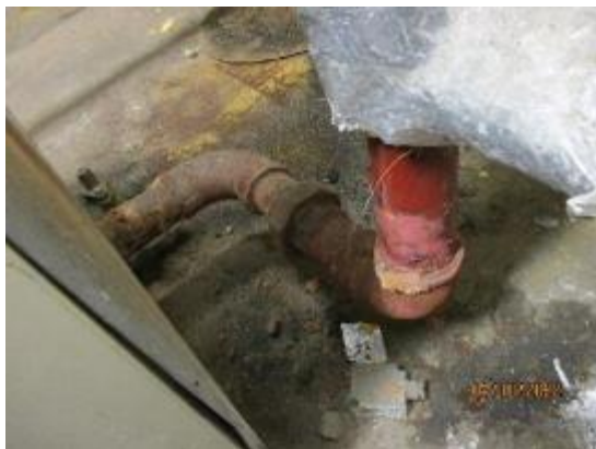
181. Pipework – heating system. Plant room 1/26
