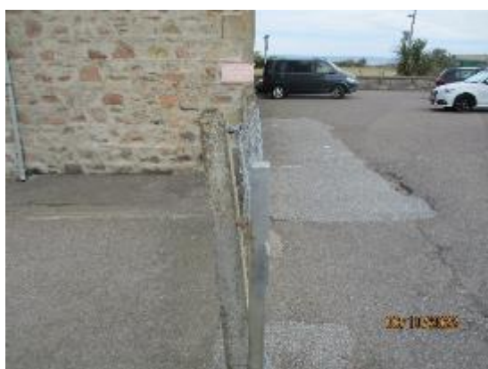
254. Leaning concrete post
