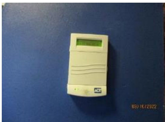
216. Intruder alarm keypad. 1/1
