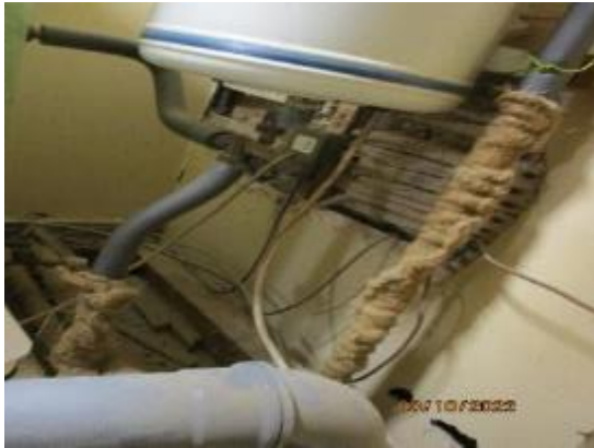
188. Pipework – hot water distribution above staff room.
