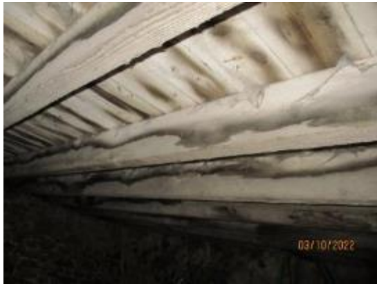
9. Watermarked roof timbers
