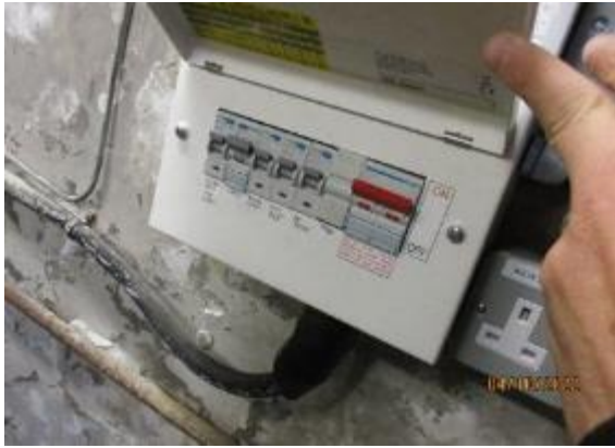
200. DB – Plant room.
