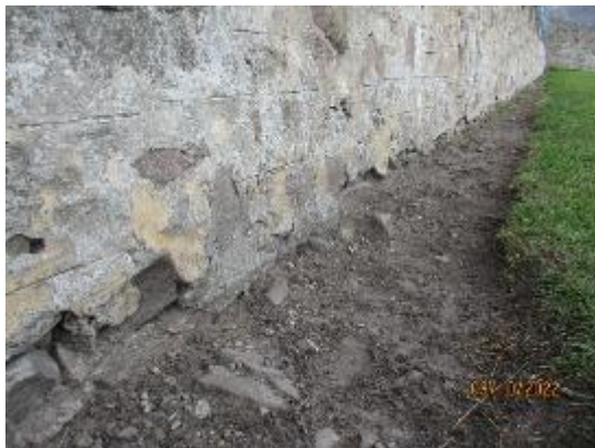
274. Erosion at ground level
