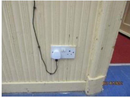
201. Flush socket – typical. Gym hall.
