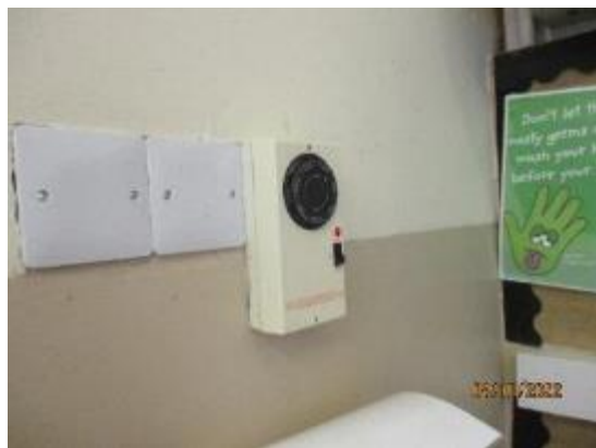
241. Heating system timeclock. Main open area.
