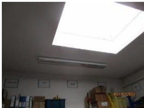
205. Office lighting typical.
