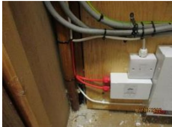
215. Fire alarm magnetic door interface and wiring. Cupboard 1/22.
