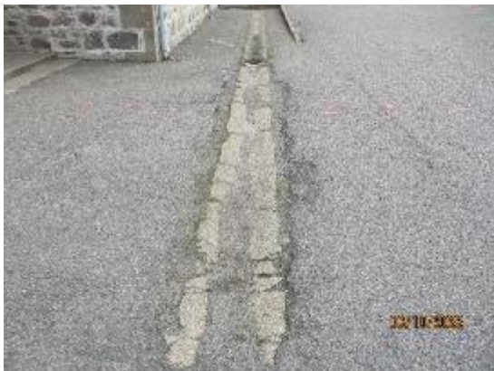
280. Broken concrete drainage channel
