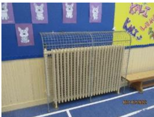
183. Radiator – gym/dining hall main school.
