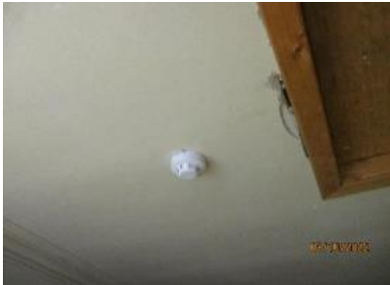
214. Fire alarm detector head. 1/11 typical.
