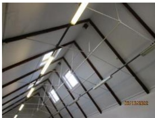
207. Lighting – gym/dining hall.
