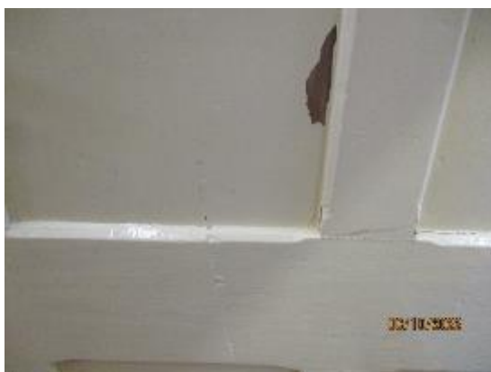
123. Damaged timber doors
