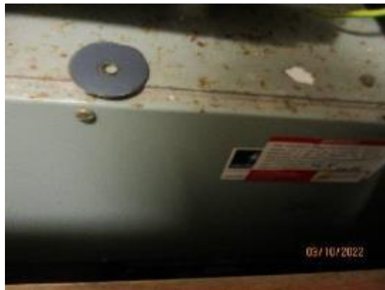
197. Main busbar. Cupboard 1/22
