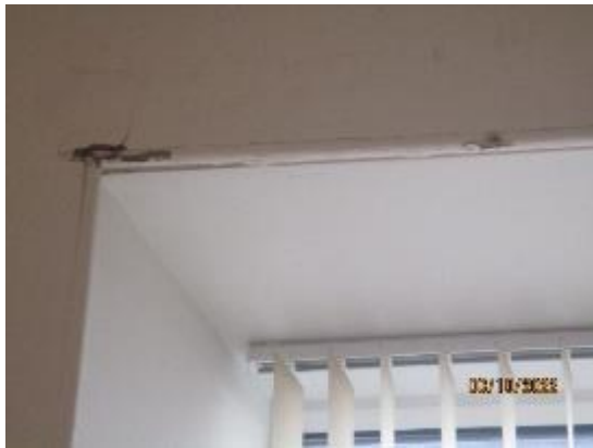
119. Damage to window linings
