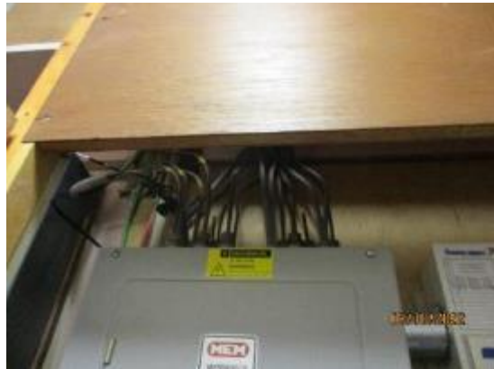
203. General wiring MICC cupboard 1/22
