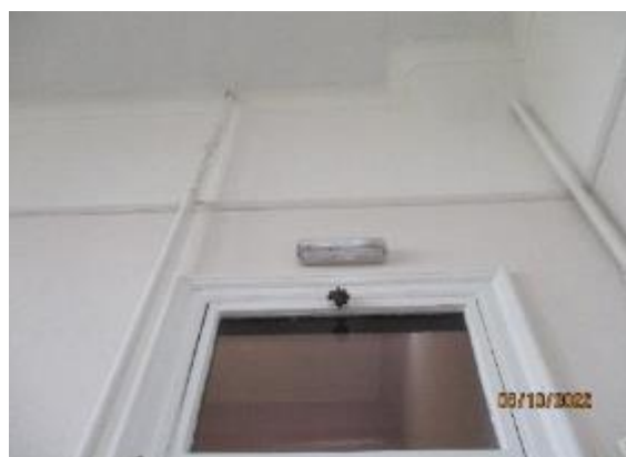
208. Emergency lights. – Library,
