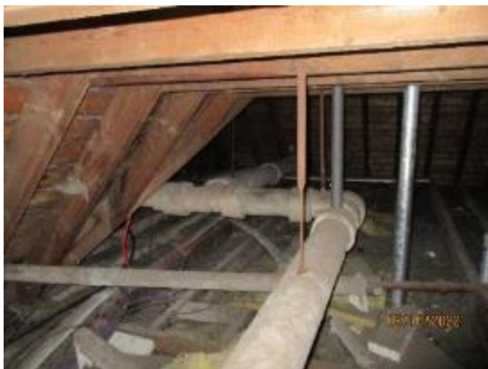
180. Heating distribution pipework – Attic space
