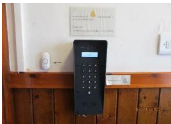
220. Security door entry intercom system with camera 1/1a
