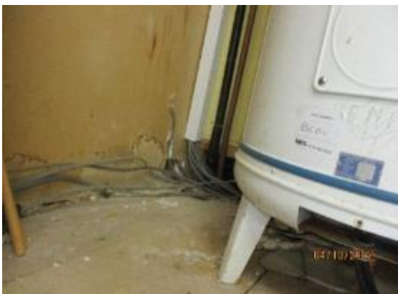
234. General wiring cupboard 1/B4
