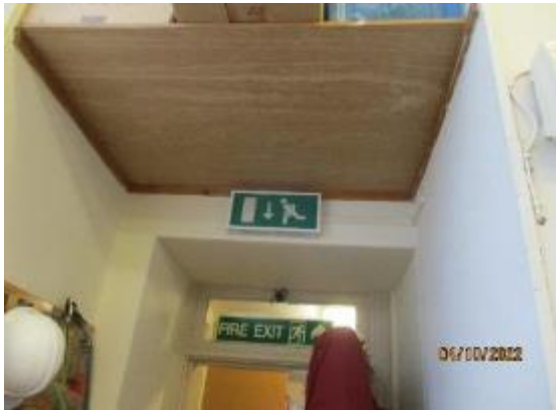
238. Emergency exit lighting. Typical.
