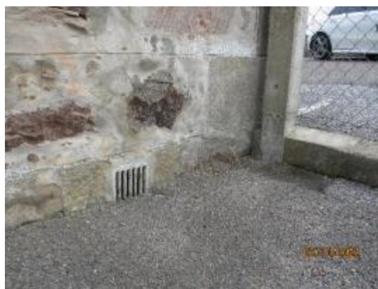
50. Ground level breaching sub-floor ventilation
