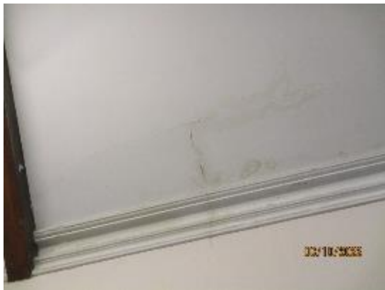
98. Lath & plaster ceilings – cracking
