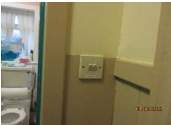
240. Lighting – control switch. Typical.
