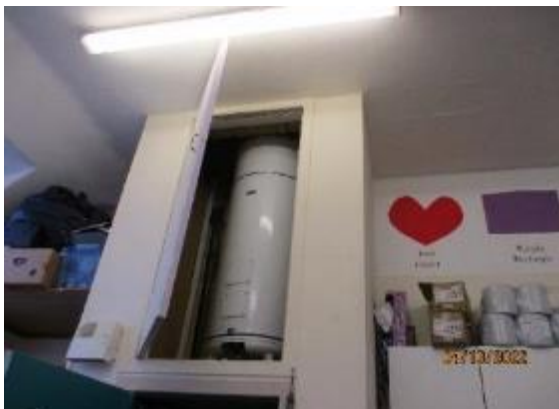
228. Hot water cylinder 1/B4 cupboard
