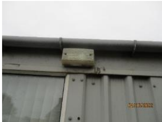
239. External building lighting. Typical.
