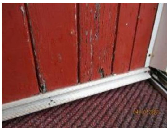
58. Wet rot in timber door to Nursery
