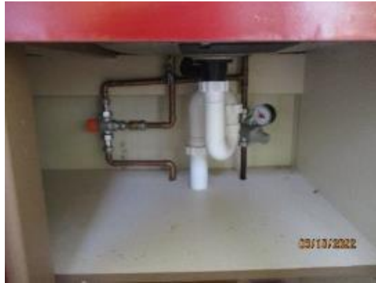
189. Pipework – hot water class 1/17 under sink.
