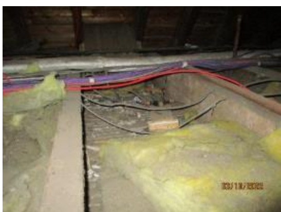
23. Thin and missing mineral fibre insulation
