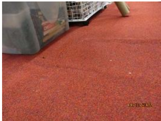
81. Eneven floor boards
