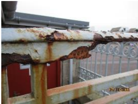
261. Corroded with sharp edges
