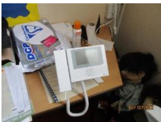
221. Security door release monitor and handset. Head teachers office 1/8
