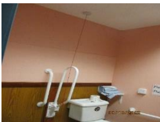
219. Disabled alarm system – pull chord 1/12
