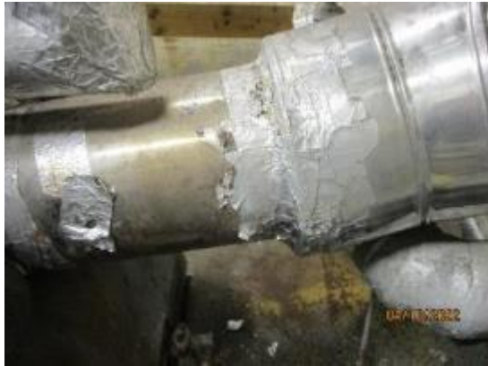
177. Boiler flue / chimney 0/26
