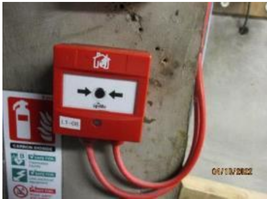
212. Fire alarm call point device. 0/26
