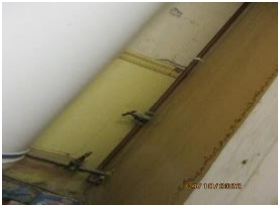
230. Cold water mains pipework. Cupboard 1/B4
