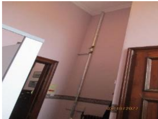
191. Cold water pipework. Entry point. 1/5 toilet.
