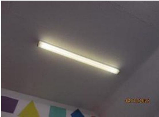
236. Lighting – main open area. Typical.
