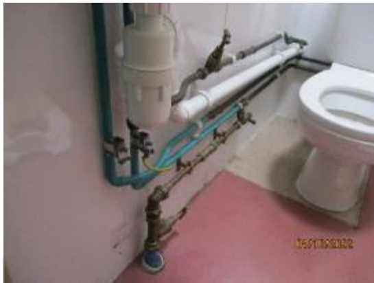
231. Cold mains pipework – cold water entry 1/B2
