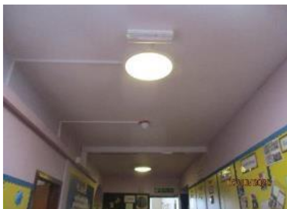
206. Lighting – access corridor. 1/1
