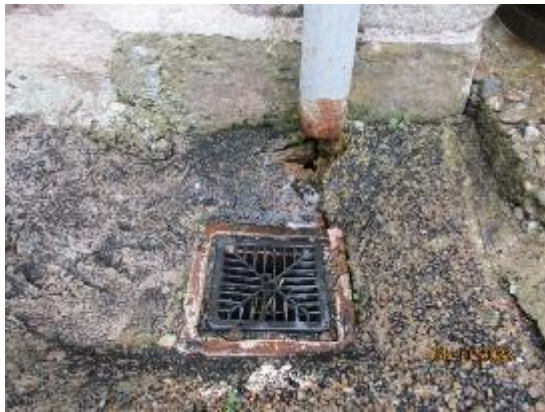
279. Cracked surround to drainage gully
