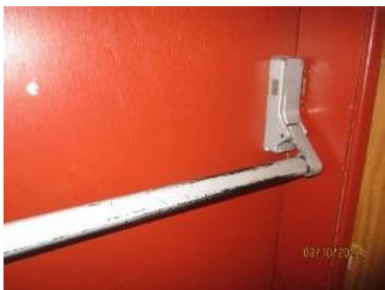
59. Fire exit panic bar ironmongery
