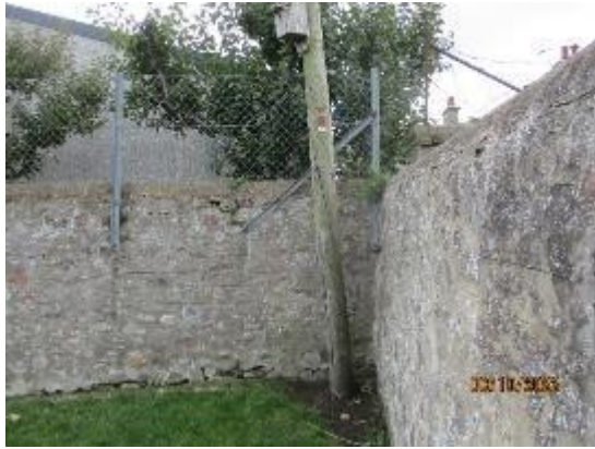
285. Leaning utility pole
