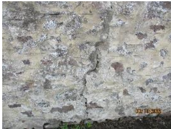
273. Cracks to perimeter wall
