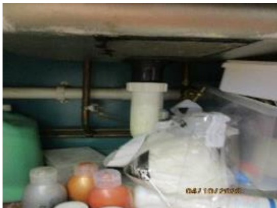
229. Hot water copper pipework under kitchen sink.
