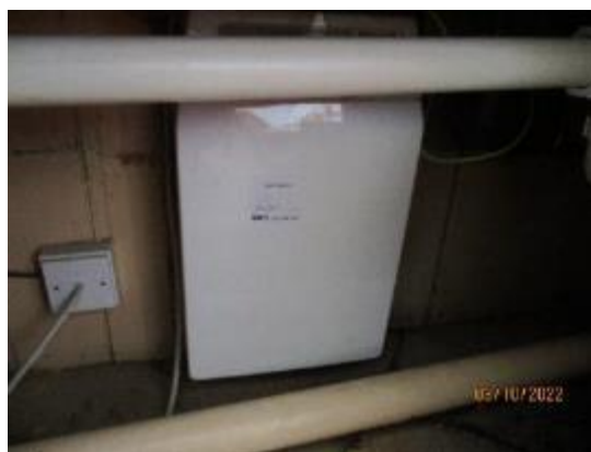
187. Classroom point of use water heater. Typical.
