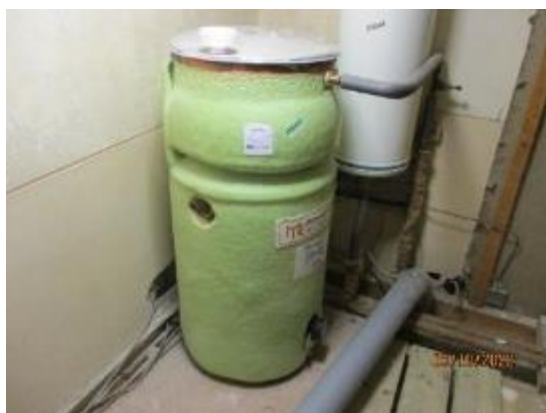
186. Hot water cylinder above staff room.
