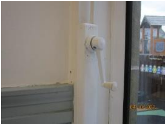
69. Faulty window winders to Nursery windows
