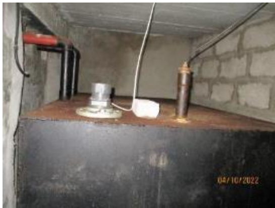
179. Oil storage tank – plant room 0/26
