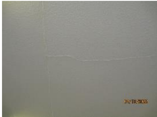
105. Cracked lath & plaster ceilings
