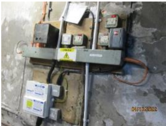
178. Heating controls plant room 0/26
