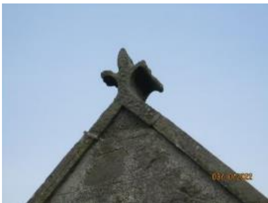
47. Stone finial – poor condition
