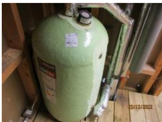
184. Hot water storage cylinder above 1/11
