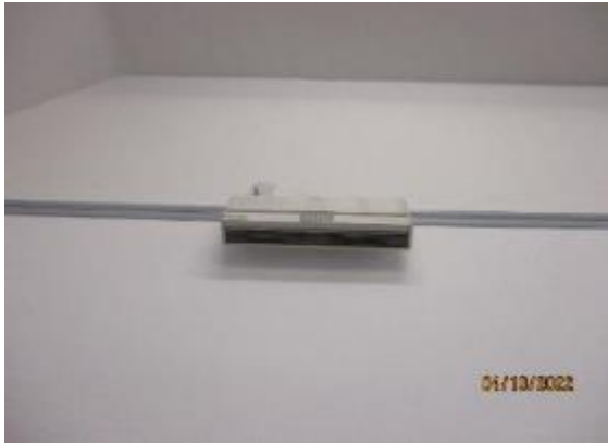
224. Electric fan convactor heater. Main classroom.
