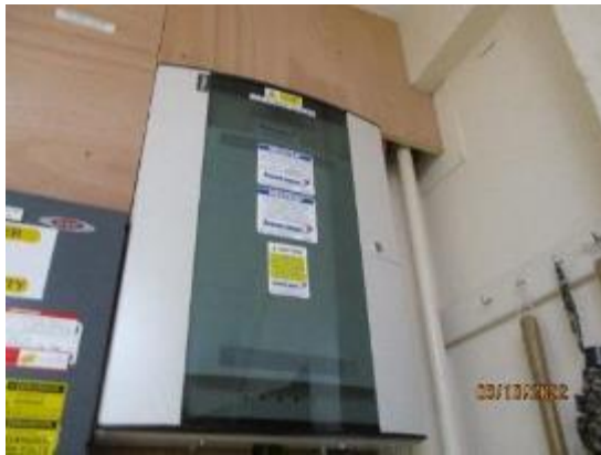
194. DB – West distribution. Janitors room 1/10
