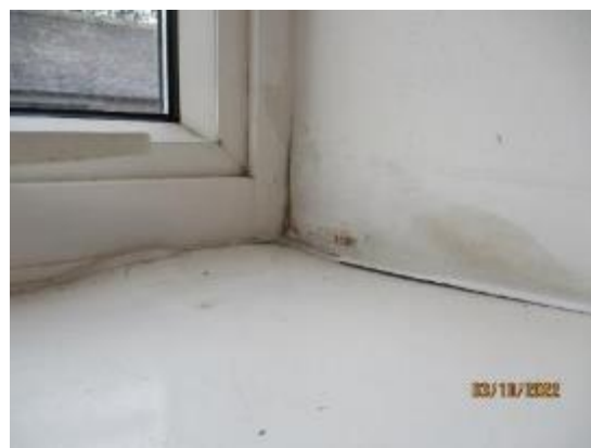
118. Window linings warped and water marked
