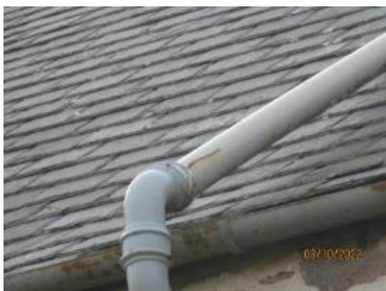
37. Cracked soil vent pipes
