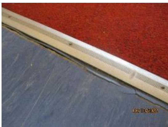
88. Linoleum cracked and worn
