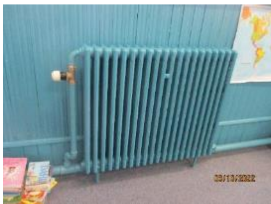
182. Radiator – Heating system. Classroom.
