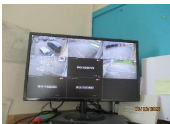
222. CCTV monitor and recorder. Reception office 1/2
