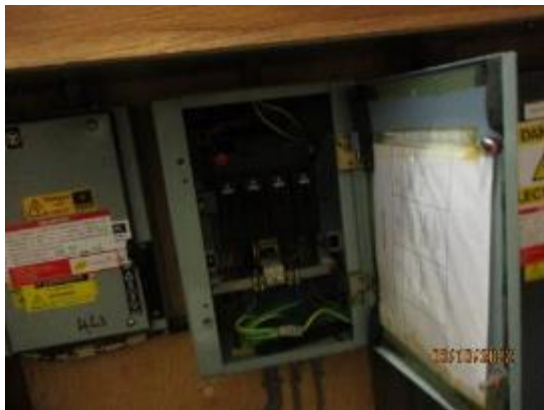
196. DB – Essential lighting cupboard 1/22
