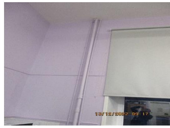
166. Pipework – heating distribution in school rooms.
