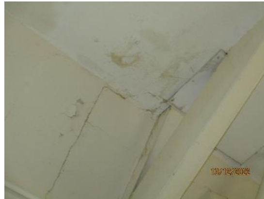
88. Water damaged ceilings
