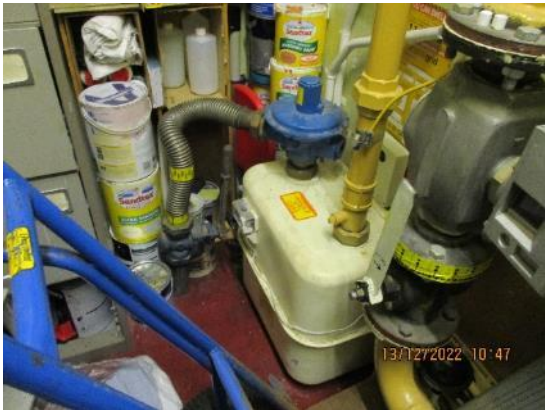
181. Gas meter and distribution pipework janitors room 1/11
