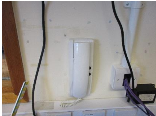
212. Security door access control handset reception office 1/1
