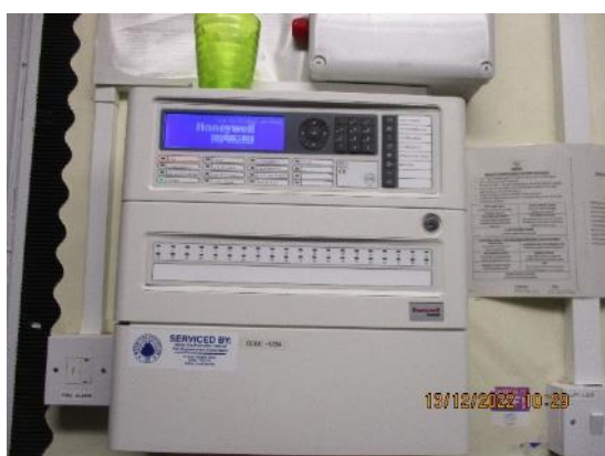
201. Fire Alarm control panel 1/12 corridor
