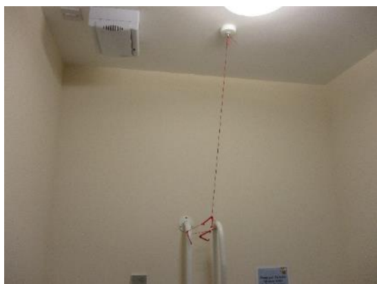
207. Disabled alarm system pull chord activation. 1/16
