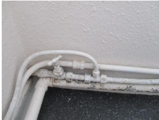
180. Pipework – cold water supply 1-18
