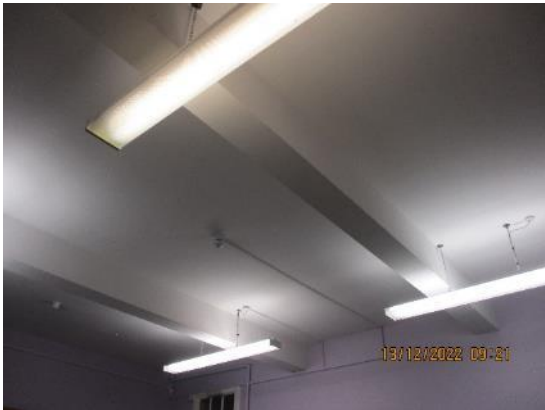
193. Lighting – classroom typical.
