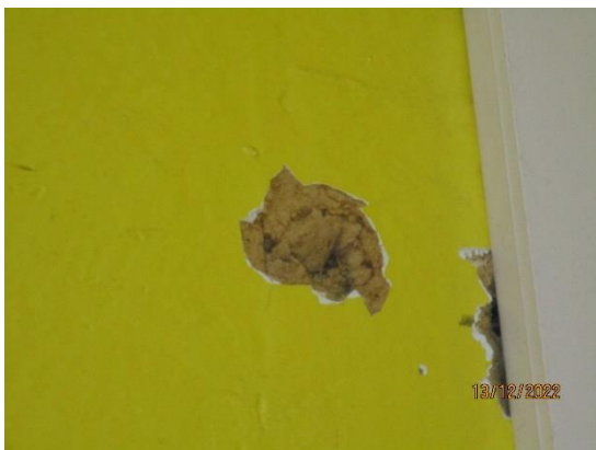
101. Damaged fibreboard walls
