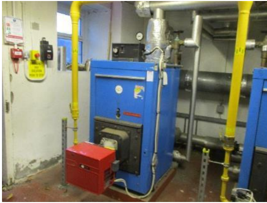
161. Boiler 1 – Plant room 0/3
