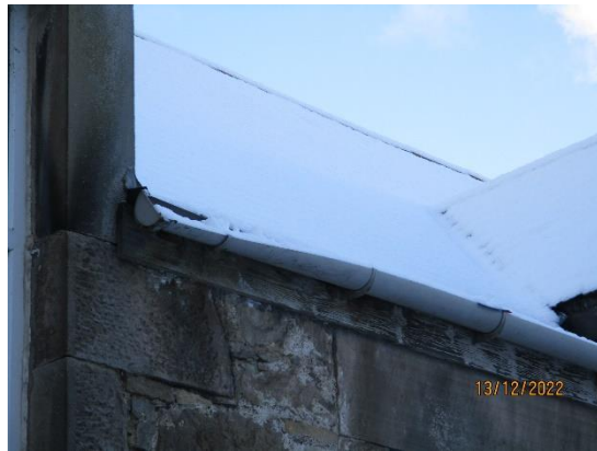
20. Collapsing UPVC gutters
