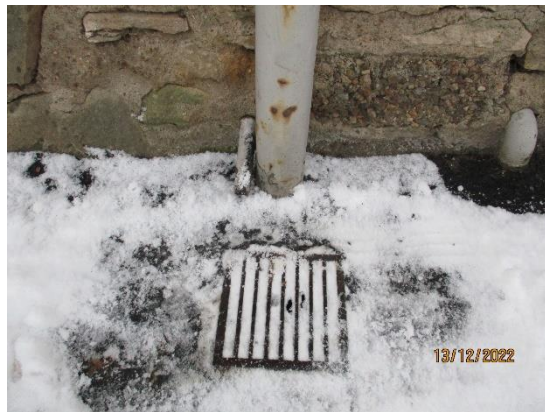
22. Back inlet gullies
