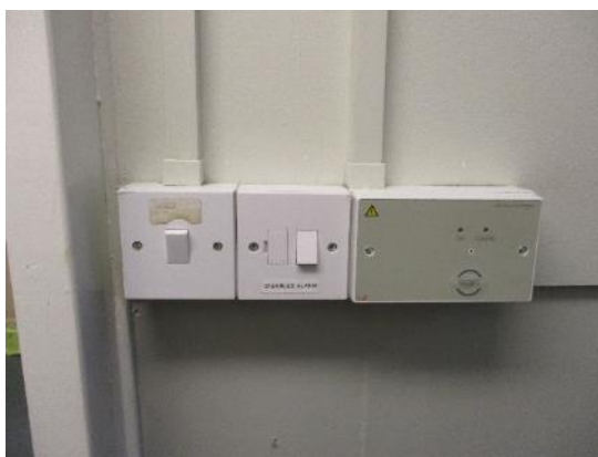
208. Disabled alarm system alert unit. 1/16
