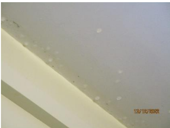
89. Condensation on underside of flat roofs
