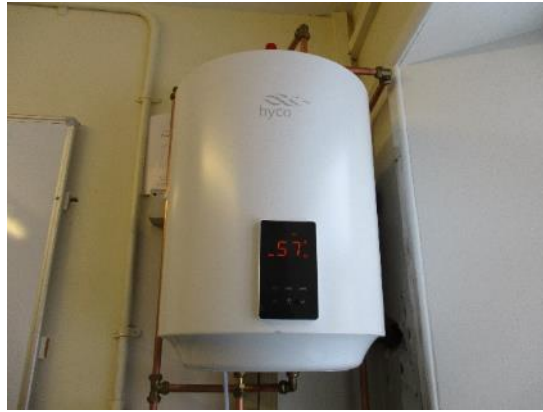
174. Calorifier – kitchen hot water storage and supply only. Located in staff room 1/20.
