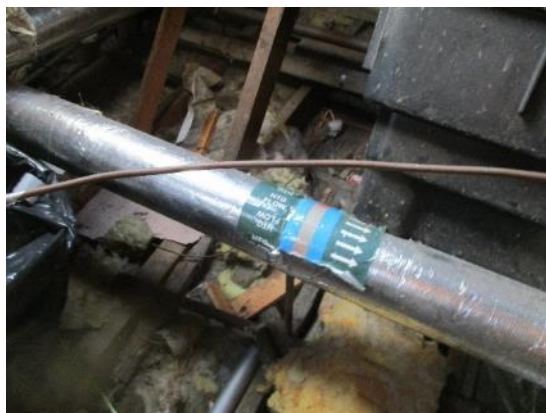
165. Pipework – heating distribution. Attic space.
