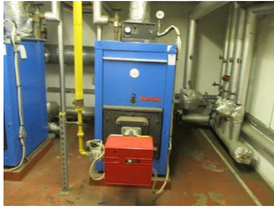
162. Boiler 2 plant room 0/3
