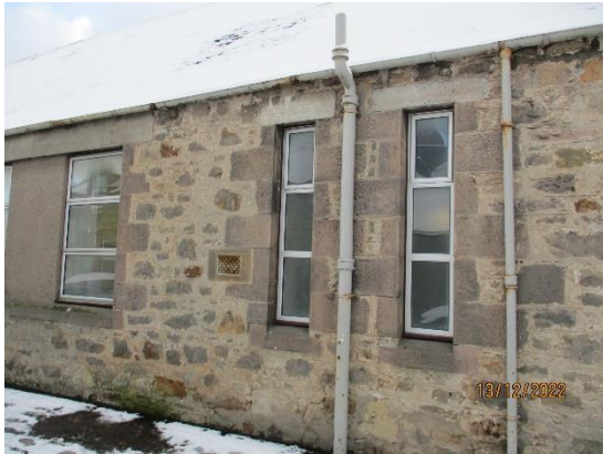
25. Cast iron soil vent pipes
