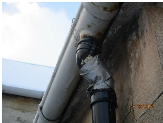
24. Damaged UPVC downpipes
