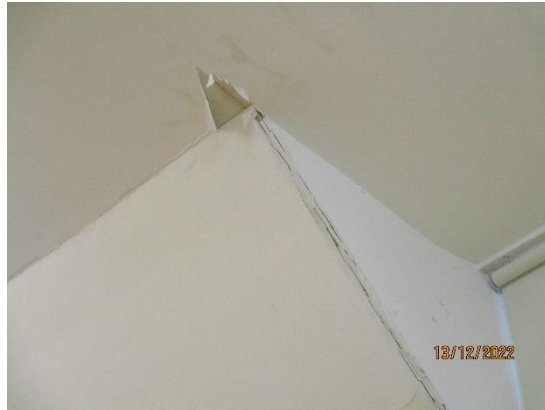
86. Cracked and damaged lath & plaster
