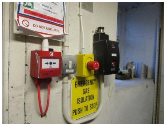
184. Gas safety supply shut off. Plant room 0/3.
