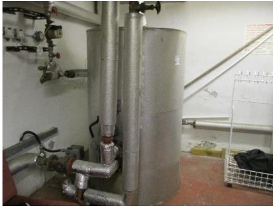
173. Calorifier. Main school hot water storage 0/3 plant room.
