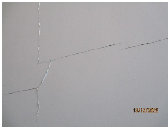
100. Cracked plastered walls
