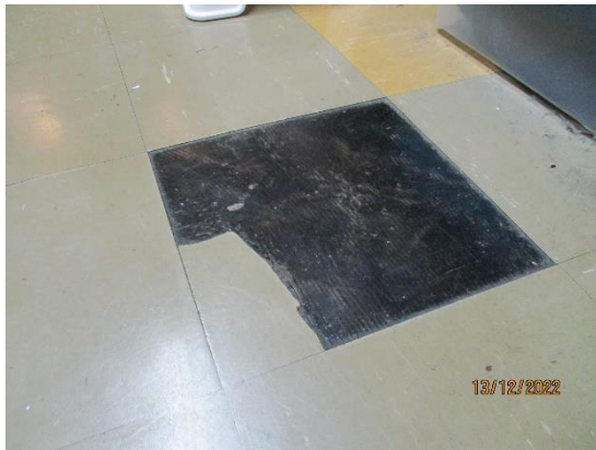
73. Missing and broken vinyo tiles
