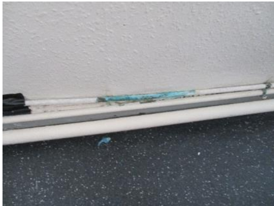
175. Pipework – hot water distribution typical.
