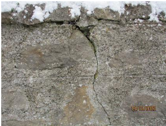
233. Pointing required to stone wall
