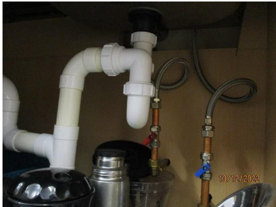
146. PVC waste pipes
