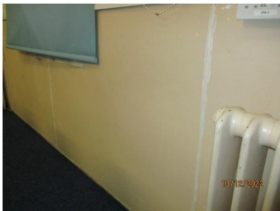
106. Wall linings – suspected asbestos
