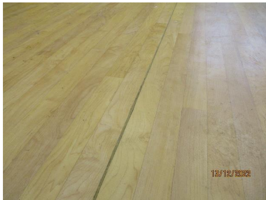
69. Open joints in vinyl flooring
