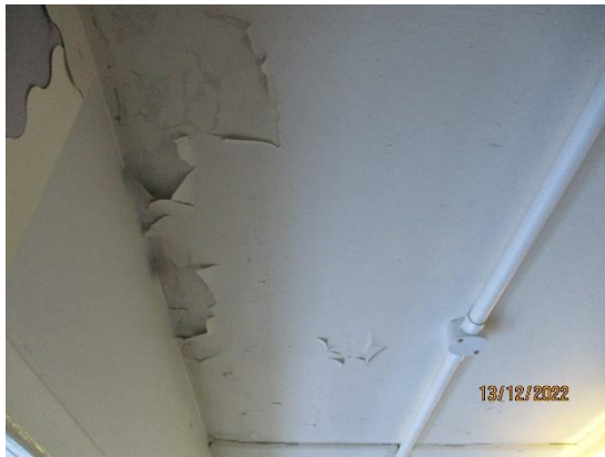
149. Ceilings – peeling paint
