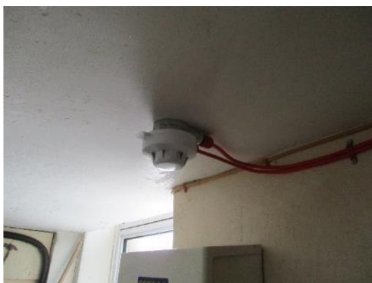
204. Fire alarm system detector and wiring typical. 1/25
