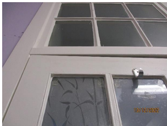
111. Twisted timber doors
