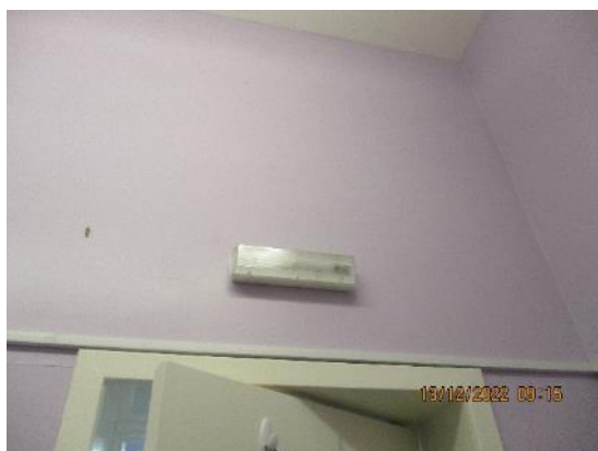
197. Emergency light fitting - classroom
