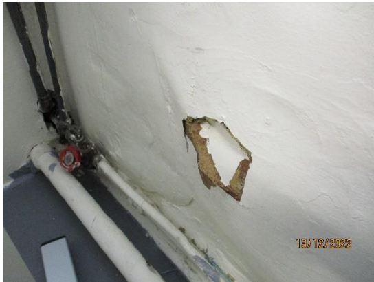
99. Damaged fibreboard walls
