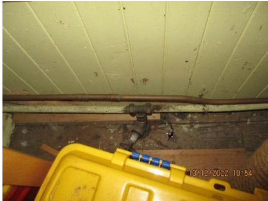
179. Pipework – cold water mains supply 1/14 typical.
