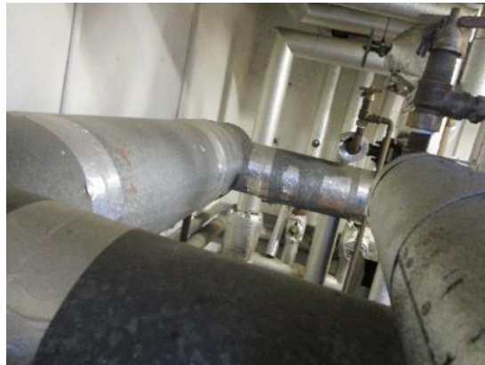
164. Flue system – boilers. 0/3 Plant room
