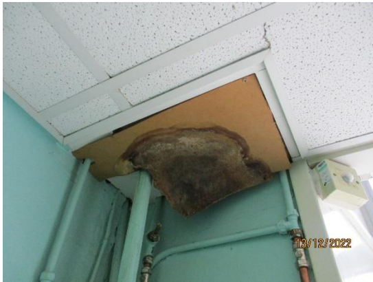
93. Water damaged suspended ceilings
