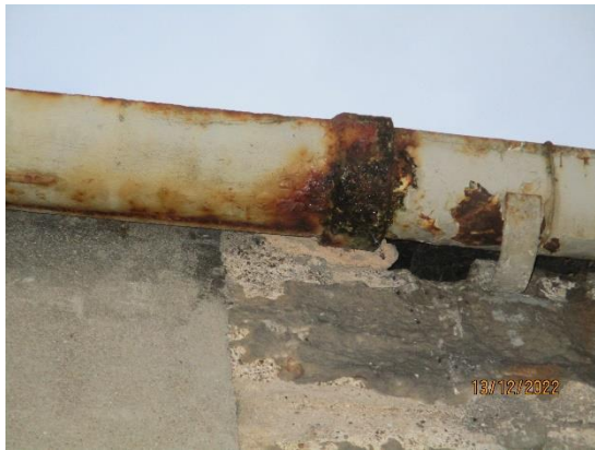
19. Leaking gutter joints
