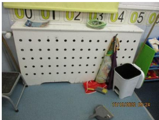
171. Radiator – nursery with protective cabinet.
