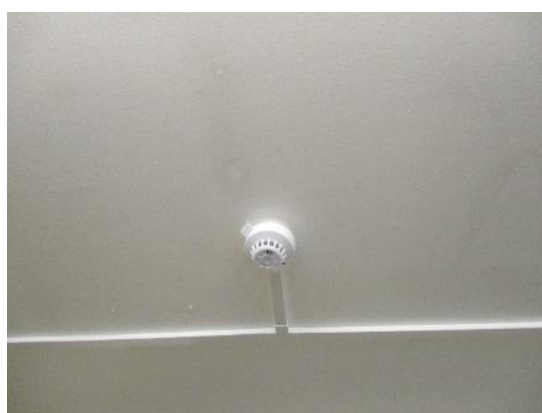
202. Fire detector head – Kitchen 1/21. Typical
