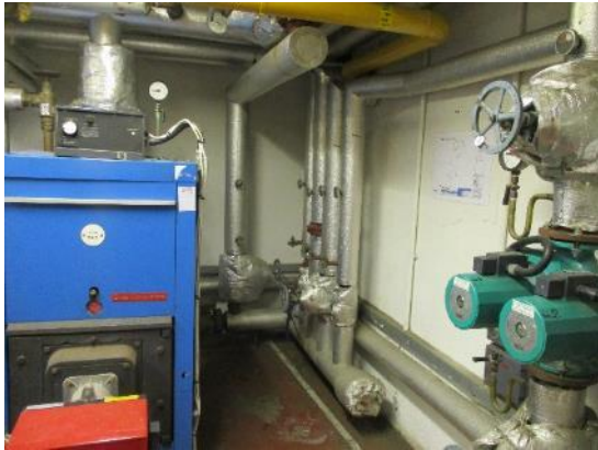
167. Pipework – heating distribution in plant room.
