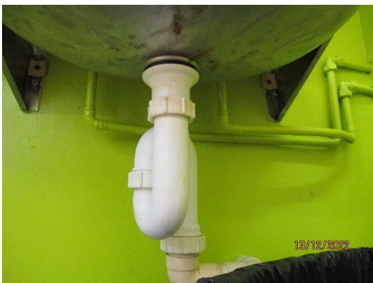
136. PVC waste pipes
