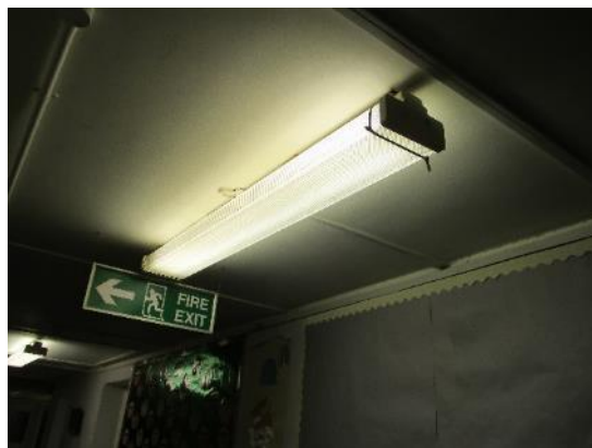
196. Lighting – corridor typical
