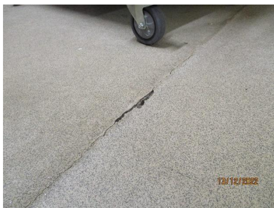
71. Cracked vinyl flooring
