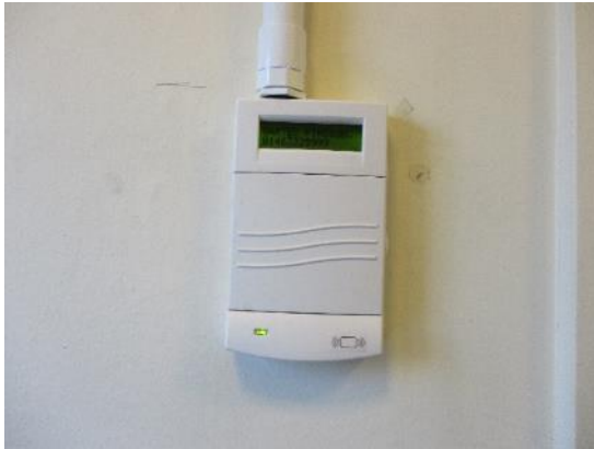
209. Intruder alarm user control unit. Main entrance 1/1
