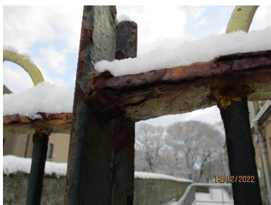
227. Corrosion of metal gates
