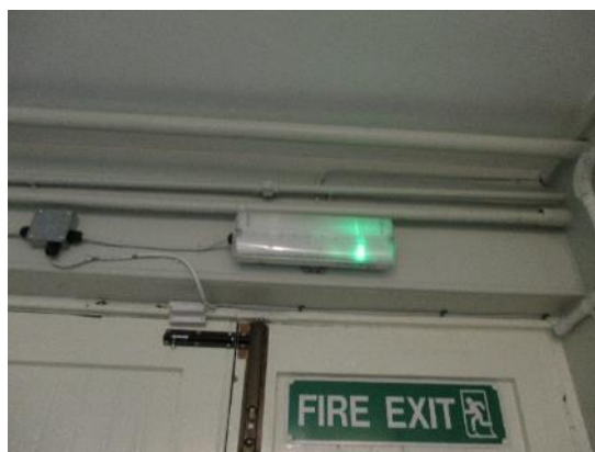
198. Emergency light. Fire exit example.
