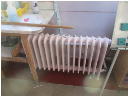
169. Radiators – cast iron section. Classroom typical.
