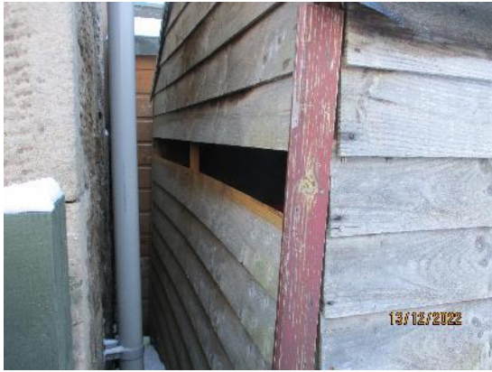
239. Timber shed – missing cladding
