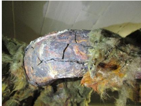
168. Pipework – heating system. Plant room.
