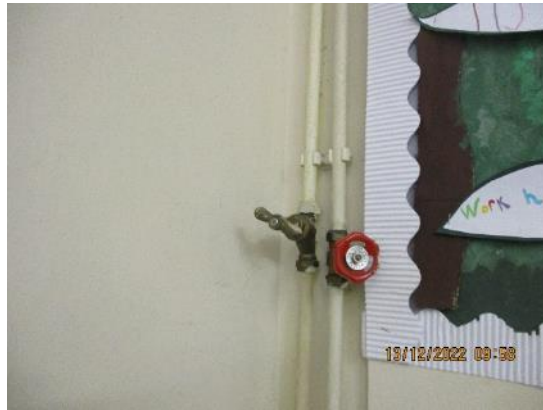
176. Pipework – hot water distribution.
