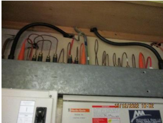
191. General wiring from DBs 1/14
