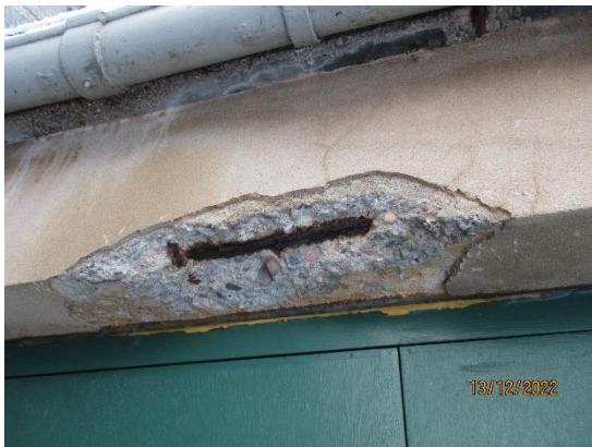
33. Spalling lintols, exposing reinforcement
