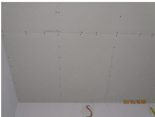
95. Plasterboard ceilings (not taped or filled)
