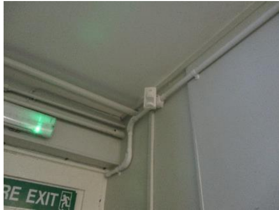
210. Intruder alarm motion sensor typical.
