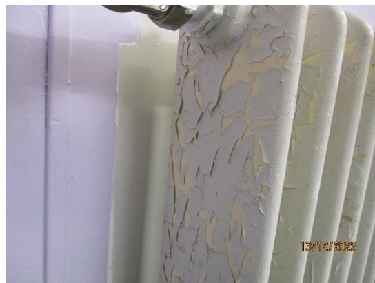
154. Cast iron radiators
