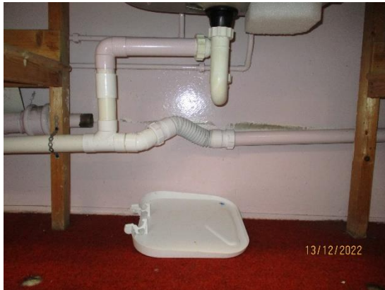
147. Poor fall on waste pipes
