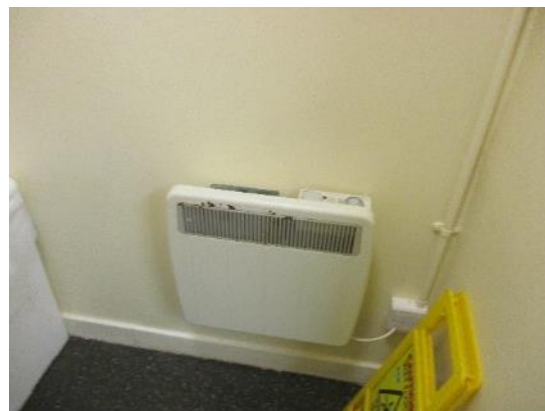
172. Electric convector heater staff toilet.
