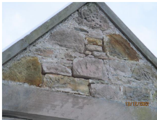
30. Isolated repointing required
