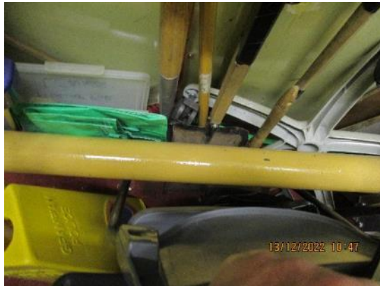
182. Gas distribution pipework room 1/11
