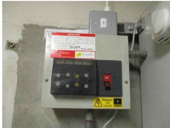
188. DB – Plant room 0/3
