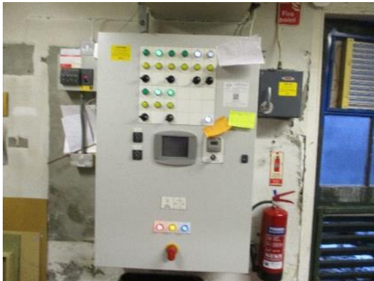
163. Control Panel – Plant room 0/3.
