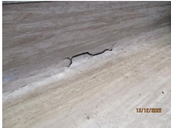
82. Torn vinyl to stairs
