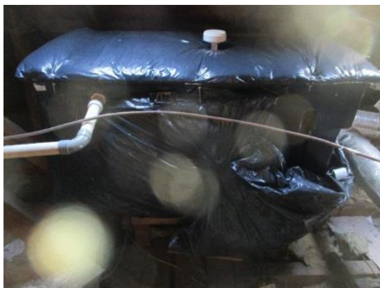
177. Cold water storage tank – attic space 2 storey part.
