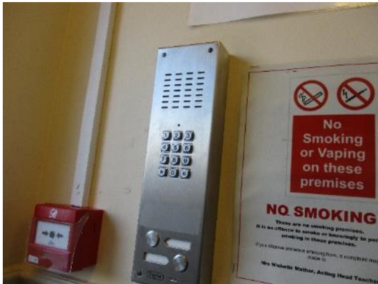
211. Security internal door access control audio and keypad unit. Main entrance 1/1
