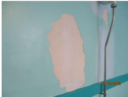
150. Walls – peeling paint
