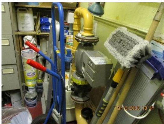
183. Gas solenoid control valve room 1/11
