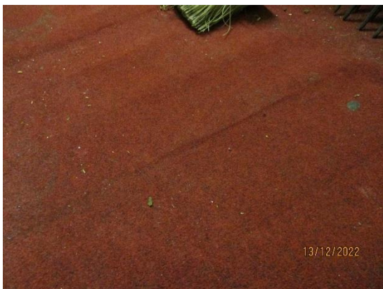
65. Uneven floor boards
