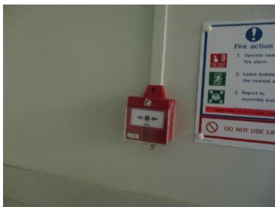
203. Fire alarm call point. Typical.
