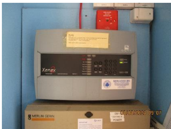
344. Fire alarm control panel – nursery building.
