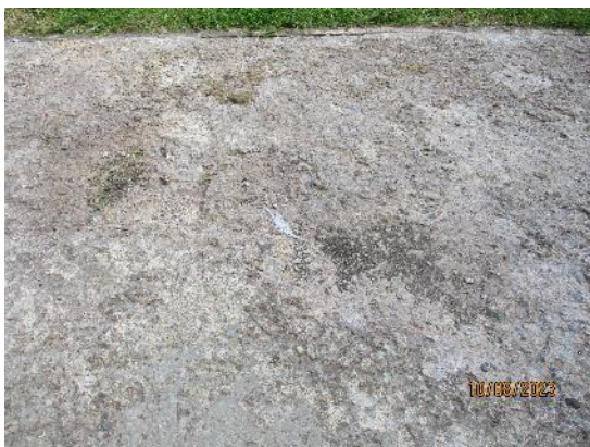
143. Eroded ramp surface
