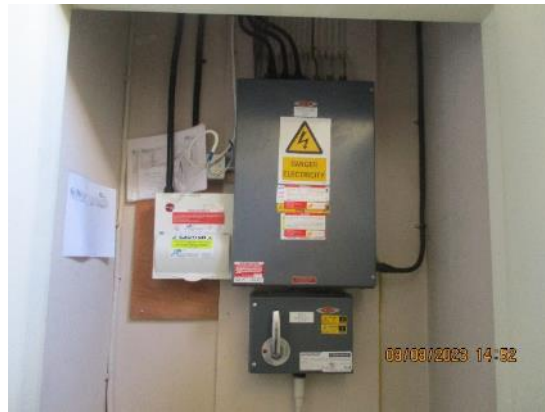
315. Distribution board – kitchen store.
