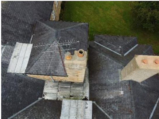
63. Open, uncapped chimney flues
