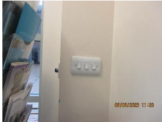
327. Light switch – 2008 extension typical.
