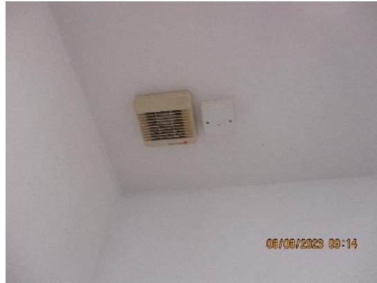
309. Extract fan staff toilet – nursery building.
