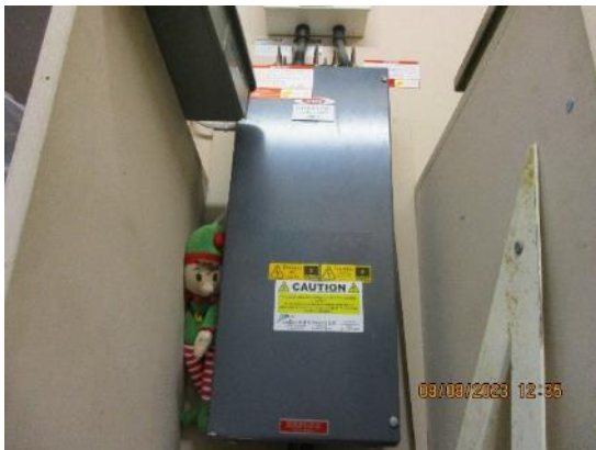
316. Distribution board – 1/37a cupboard.
