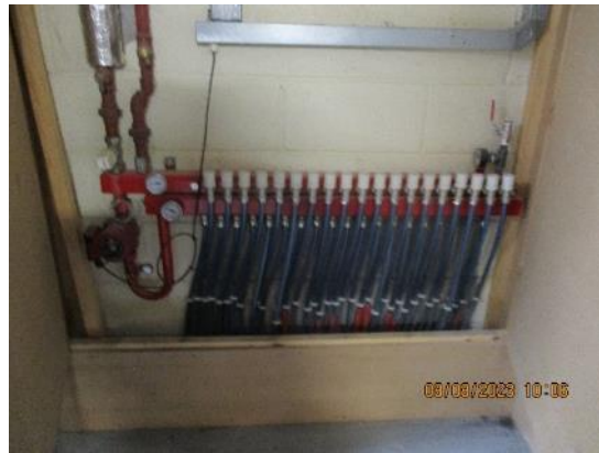
279. Underfloor heating – extension hall 1/77.
