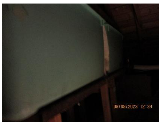
295. Cold tanks 1 and 2 above 1/37a.
