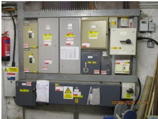
314. Main busbar and incoming power basement.
