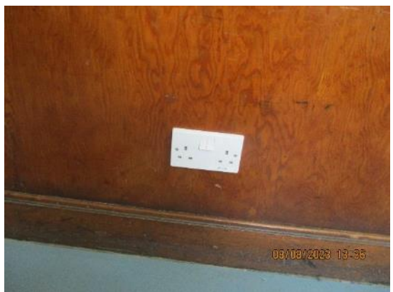
324. Flush socket – original school typical.
