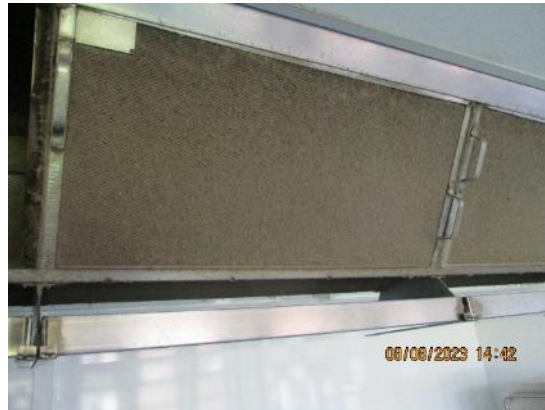
311. Kitchen extract system – filter bank (no canopy).
