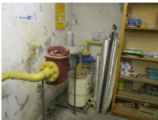
300. Gas supply pipework and meter – school basement
