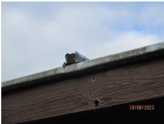
33. Missing sections of zinc
