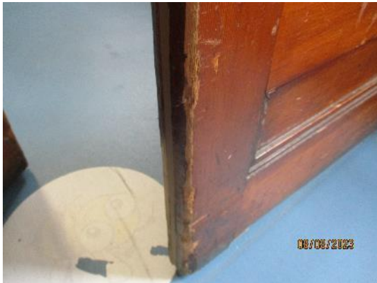
205. Damage to doors
