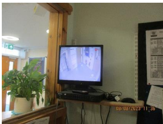
357. CCTV monitor and recorder 1/72.
