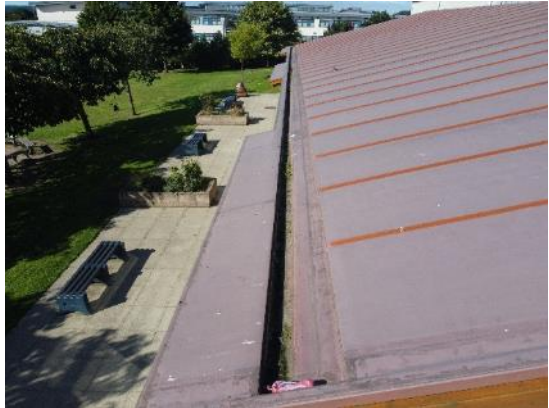
52. Single ply membrane secret gutters
