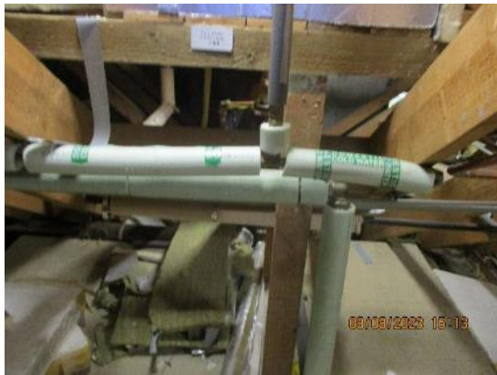
296. Cold water pipework – main school attic.
