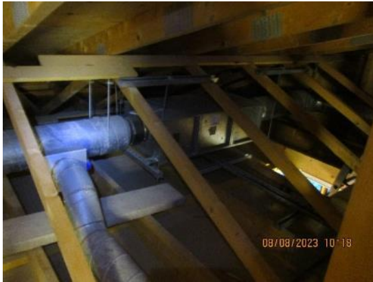
308. Centralised ventilation system ductwork 2008 extension attic space.
