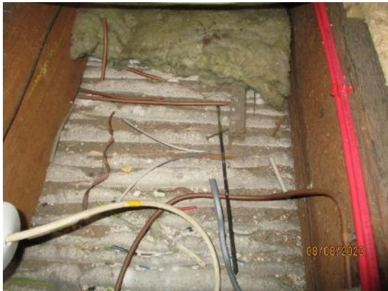
45. Insulation missing in isolated areas
