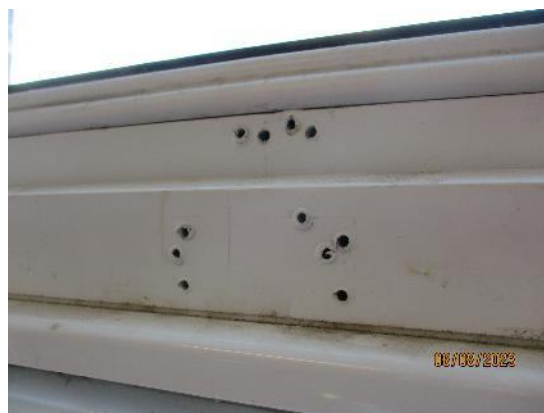
132. Missing window ironmongery
