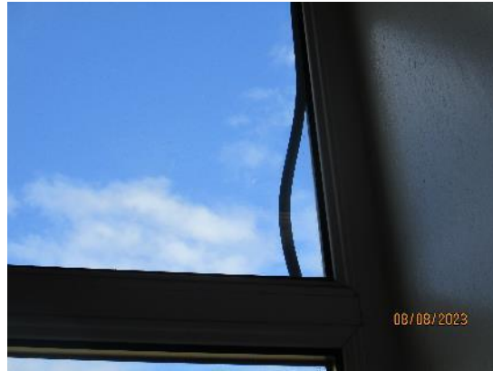
110. Failed window seals
