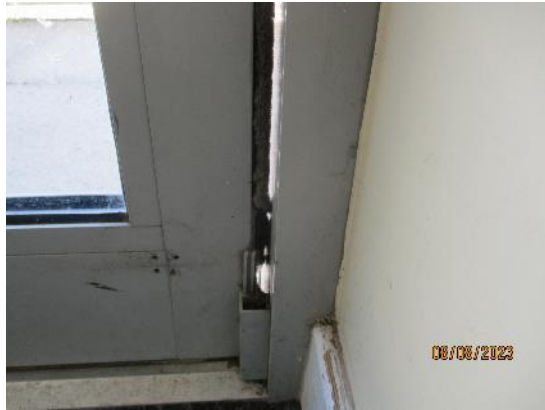
104. Gap between door and frame
