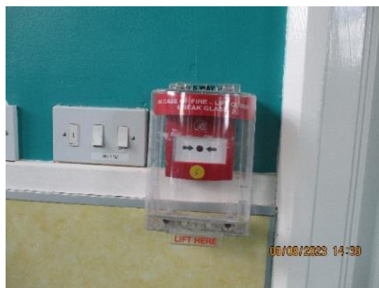
349. Fire alarm call point original school hall.
