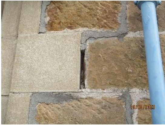
73. Isolated repointing required
