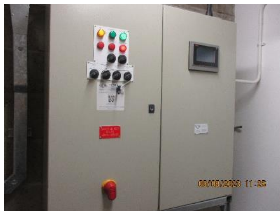
283. Heating and ventilation control panel 2008 extension.
