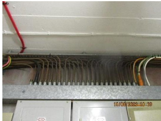
321. General wiring – basement distribution boards.
