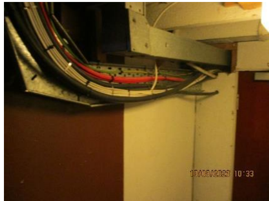
323. General wiring exiting basement boilerhouse.
