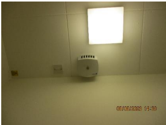
304. Extract fan – main school staff toilet.1-25a
