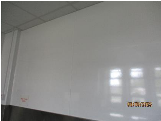
193. Wetwall to Kitchen
