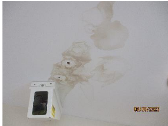
177. Water damaged plasterboard
