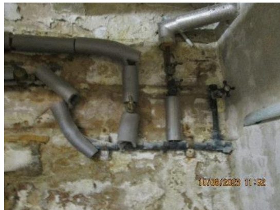
299. Cold water pipework – school basement.
