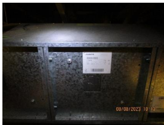
307. Centralised ventilation system unit (2) 2008 extension attic space.
