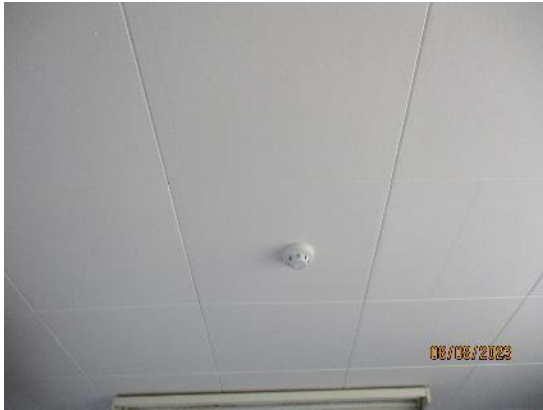
174. Asbestos ceiling tiles
