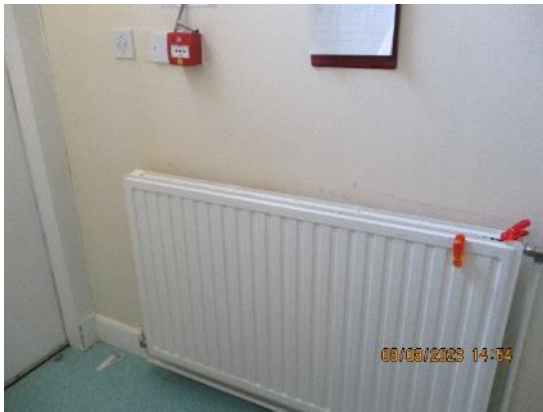
278. Steel panel radiator main kitchen corridor.
