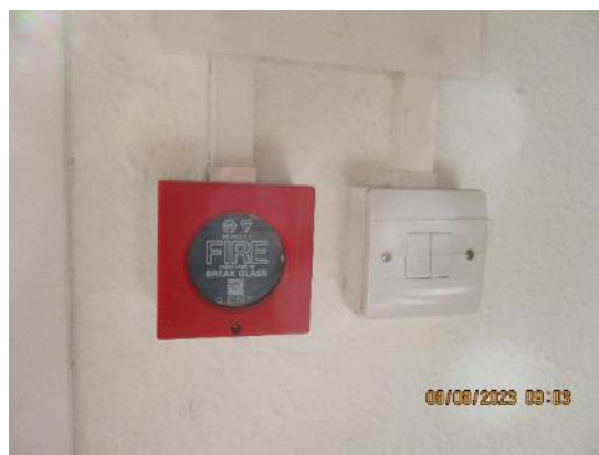
345. Fire alarm call point – nursery building.
