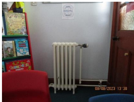
277. Cast iron radiator – original school typical.
