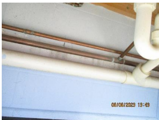
290. Hot water pipework 1975 extension.
