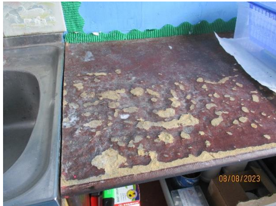
265. Water damaged worktops
