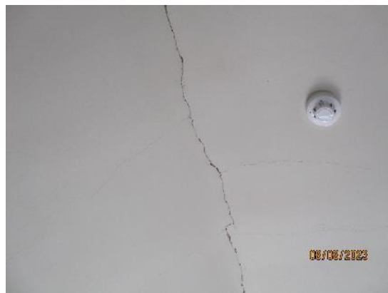
179. Cracked lath & plaster
