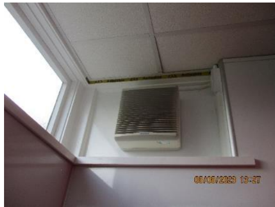
305. Extract fan boys toilet 1-35. – Main school.
