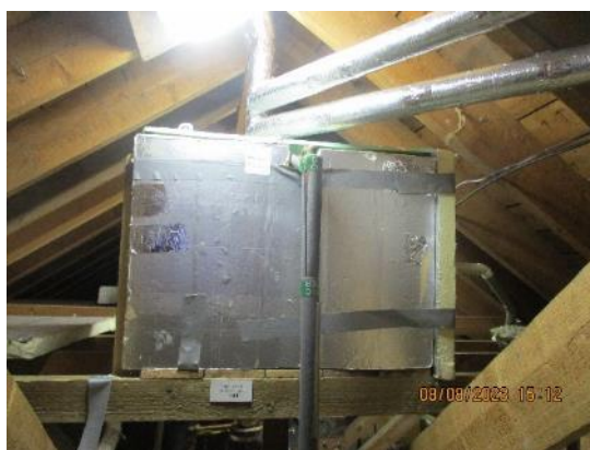
293. Cold water tank attic above 1/30. - Main school.
