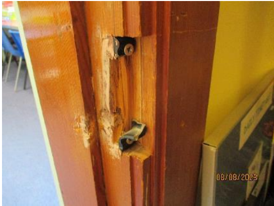
203. Damage to door frames
