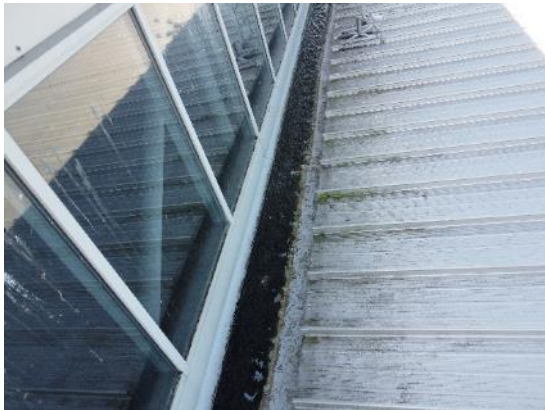
57. Blocked with silt
