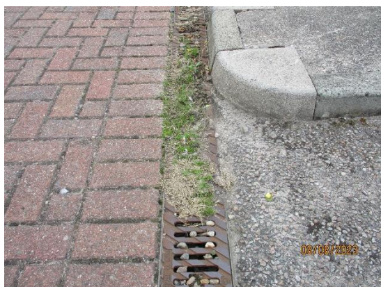
397. Car park drainage channel blocked
