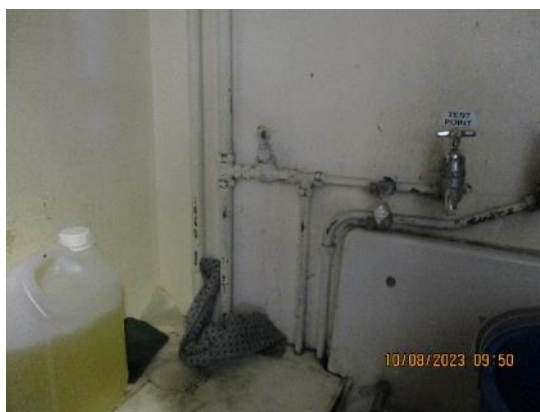
291. Hot water pipework – original school.
