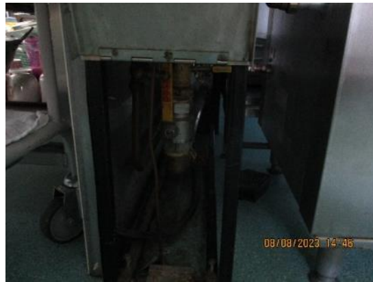
303. Gas pipework behind cooking appliances - kitchen.
