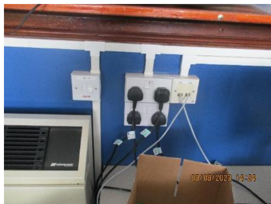
325. Sockets computer room 1/18.
