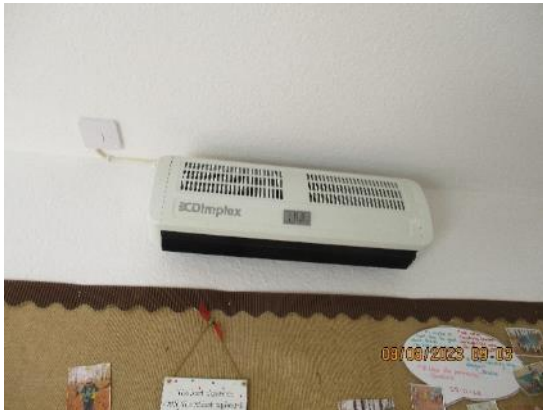
280. Electric fan heater – nursery building.
