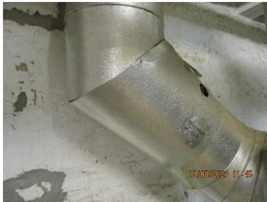
273. Boiler steel flue into brick chimney.
