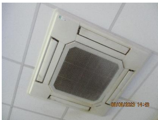
313. Air conditioning unit (1 of 2) Kitchen.
