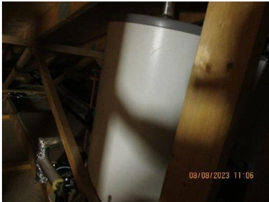
286. Hot water cylinder (1 of 2) 2008 extension attic.
