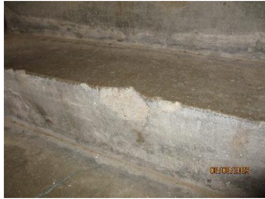
164. Chipped nosings to basement
