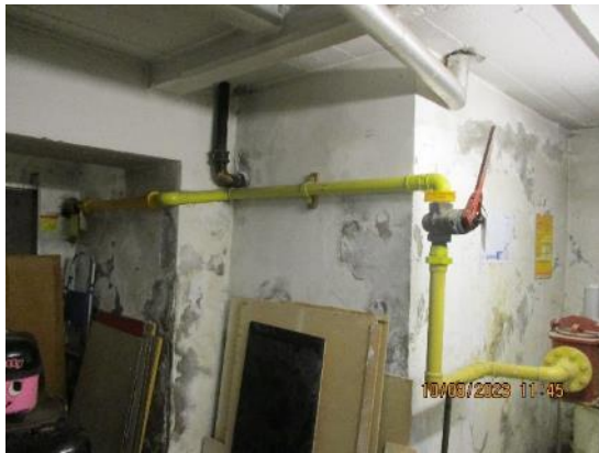
302. Gas pipework incoming to basement - main school.
