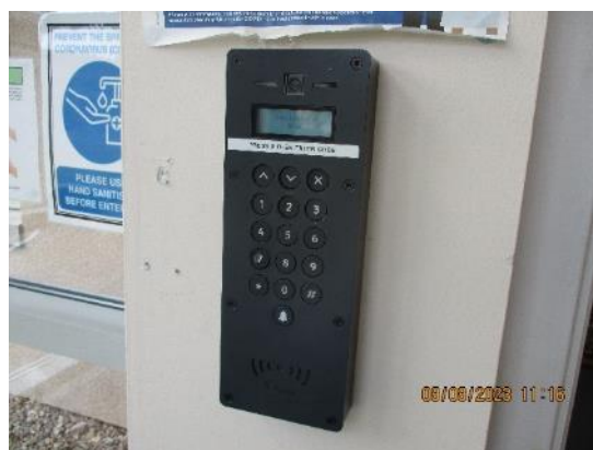
353. Door access unit – 2008 extension 1/71
