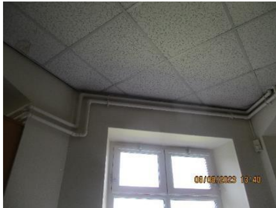
275. Heating pipework – main school.
