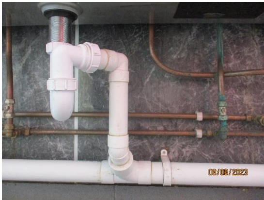
233. UPVC waste pipes
