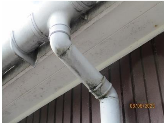
62. UPVC downpipes leaking at joints
