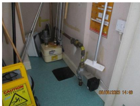
301. Gas pipework and solenoid valve - kitchen store.
