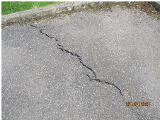
371. Tarmacadam paths cracked by tree roots
