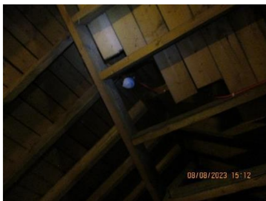
348. Smoke detector original school attic space.
