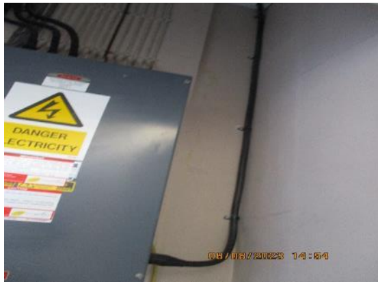
320. Sub mains cabling 1/42e original school.
