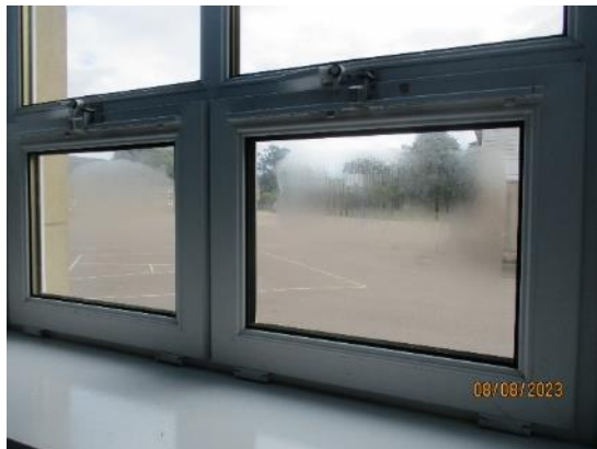
129. Failed double glazing units
