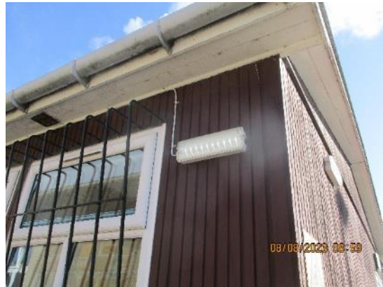
341. External lighting – nursery building.
