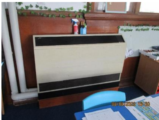
276. Fan convactor heater – classroom typical.
