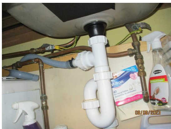
251. UPVC waste pipes to classroom sinks
