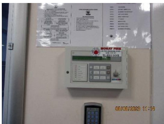
346. Fire alarm repeater panel 2008 extension 1/71.
