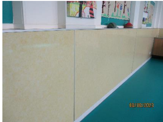
194. Wetwall in Hall
