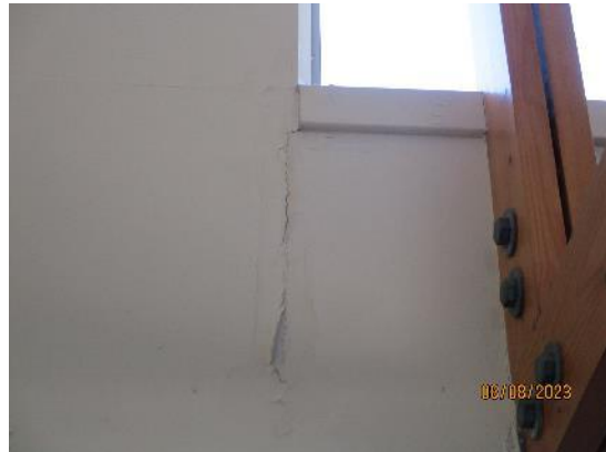
188. Water damaged plasterboard
