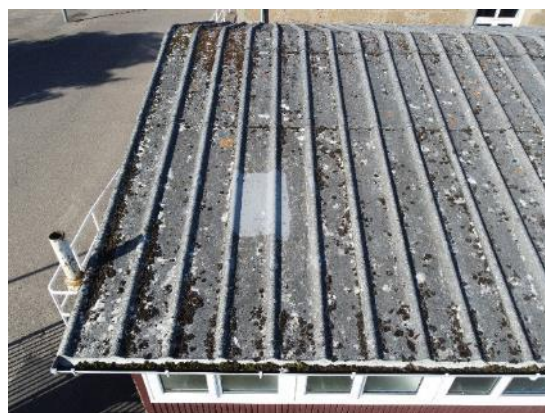
35. Surface erosion and previous repairs
