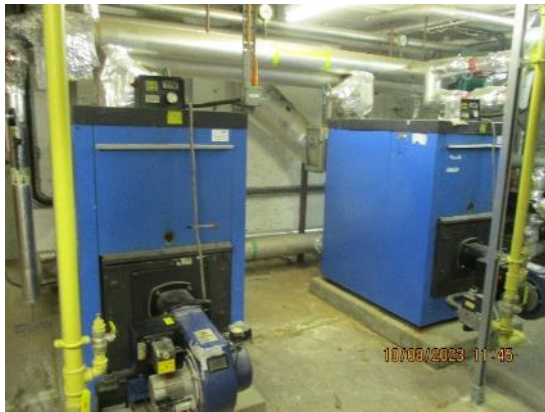
272. Natural gas boilers main school basement.
