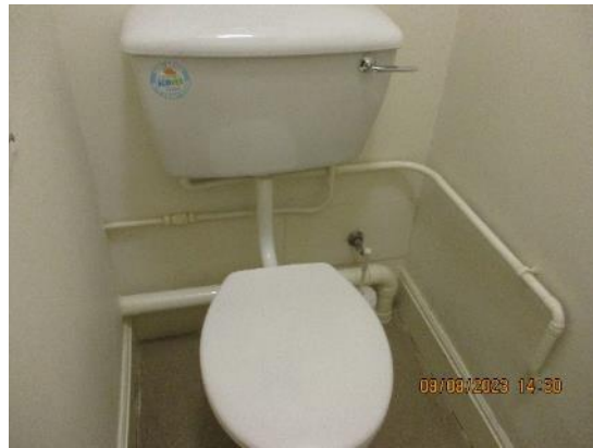
297. Cold water pipework - toilet 1/25a.
