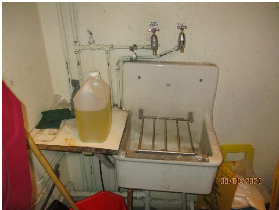
247. Cleaners Butler sinks
