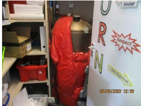
285. Hot water cylinder – main school 1/37a cupboard.
