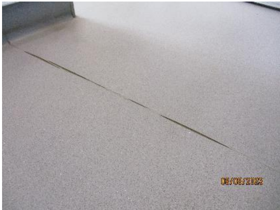
153. Open joints in vinyl flooring
