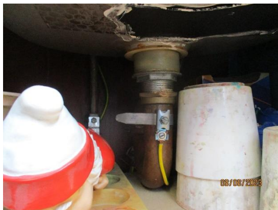
250. Copper waste pipes to classroom sinks
