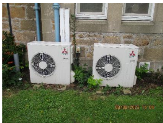
312. Air conditioning outdoor units – kitchen.
