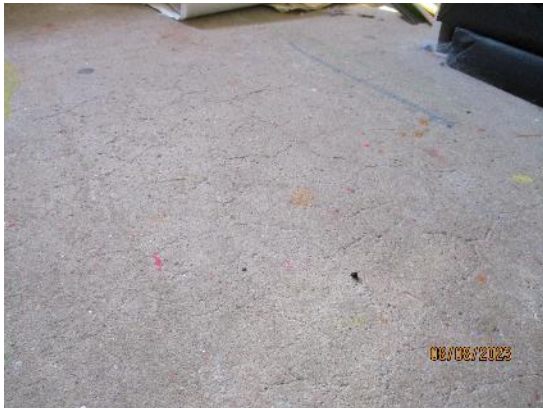
147. Concrete floors with hairline cracking
