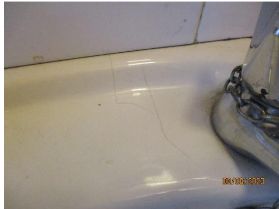
230. Hairline cracks in basins
