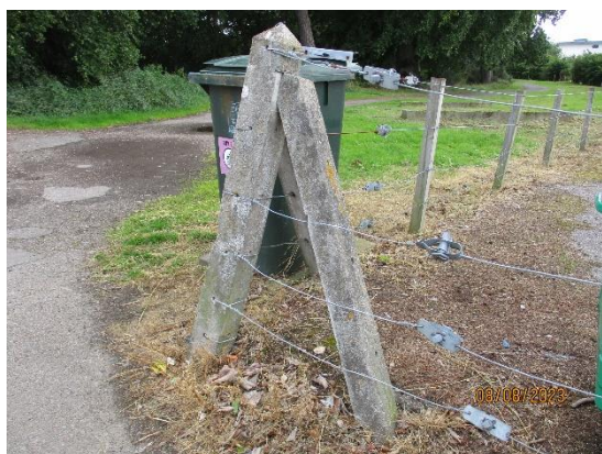
385. Impact damage to concrete posts
