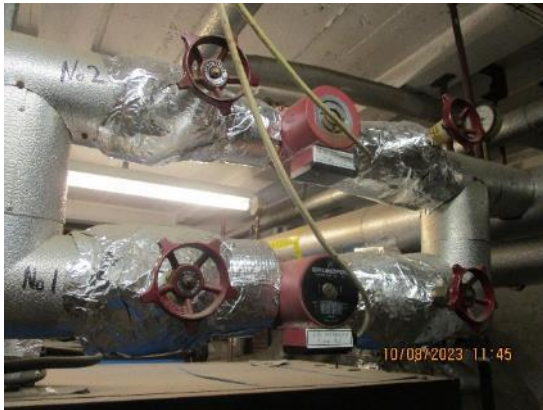
274. Heating system pipework – boilerhouse.
