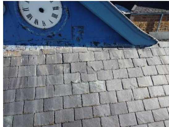
16. Isolated broken and slipped slates
