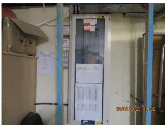
318. Distribution board – 2008 extension gym store.
