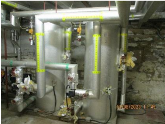
284. Calorifiers 1 and 2 – school basement.
