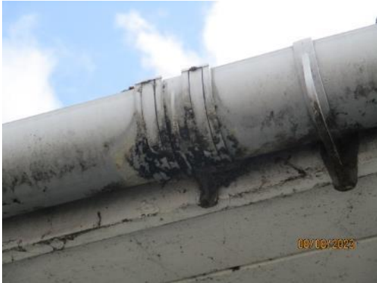
51. UPVC gutters leaking
