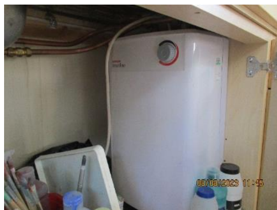
288. Point of use electric water heater 2008 extension.
