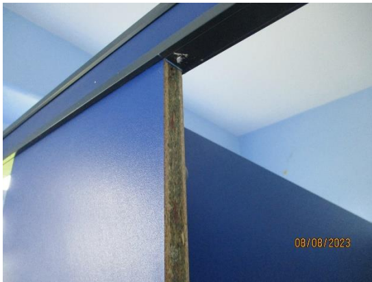
239. Missing edging strips
