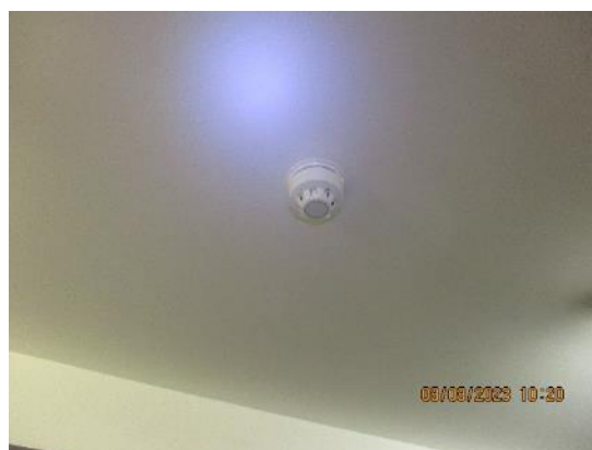
347. Smoke detector 2008 extension typical.
