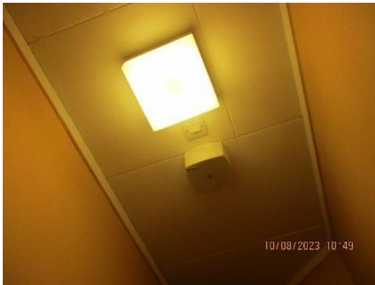
332. Lighting – original school toilet typical.
