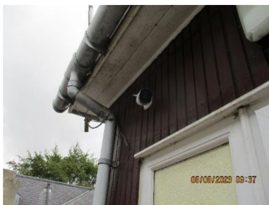
359. CCTV – Wi-Fi – nursery building.
