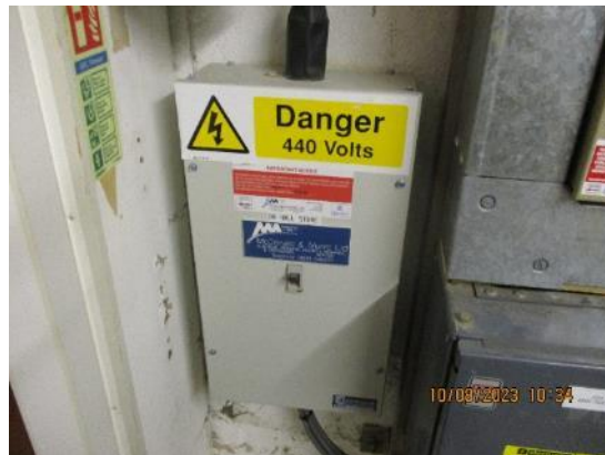
317. Distribution board hall store – basement.
