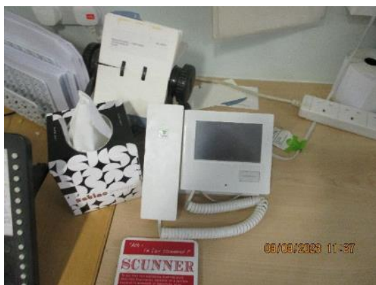
354. Door access user control handset and monitor 1/72
