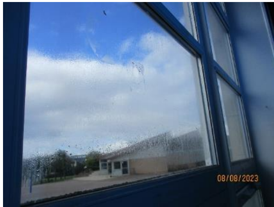
127. Condensation within double glazing
