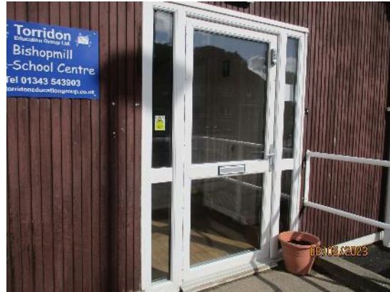
92. Single UPVC doors to Nursery
