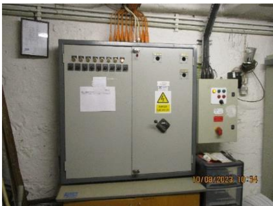
282. Heating control panel – school basement.
