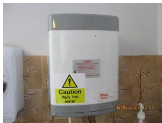
289. Point of use water heater - main school classroom.
