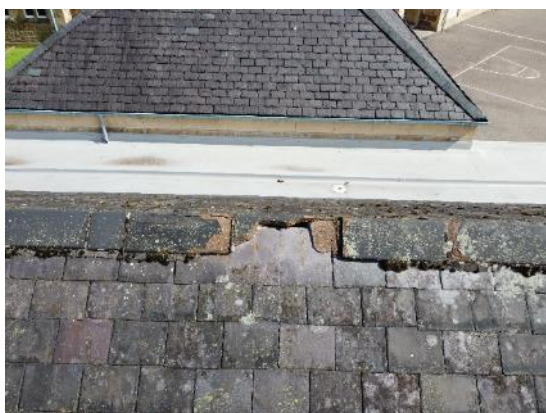
36. Damaged clay ridge tiles
