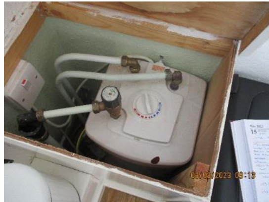
287. Point of use electric water heater – nursery.
