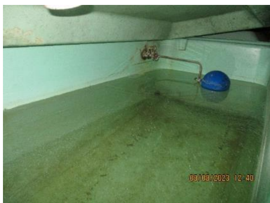
292. Cold water tank attic above 1/37a. - Main school.
