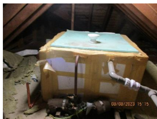
294. Cold water tank – kitchen cold supply main school.
