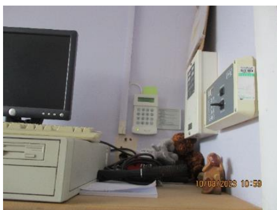
350. Intruder alarm keypad – office 1/3.
