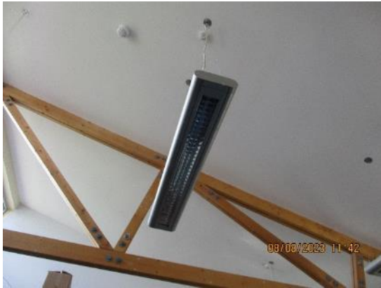
338. Lighting – 2008 extension classrooms.
