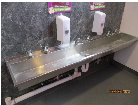
231. Stainless steel trough basins in 1975 extension
