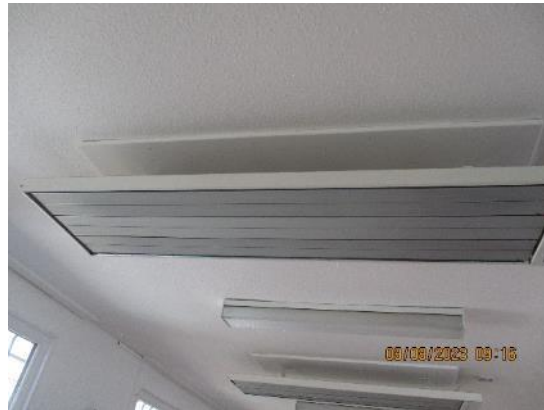
281. Electric radiant panel ceiling heater – nursery.
