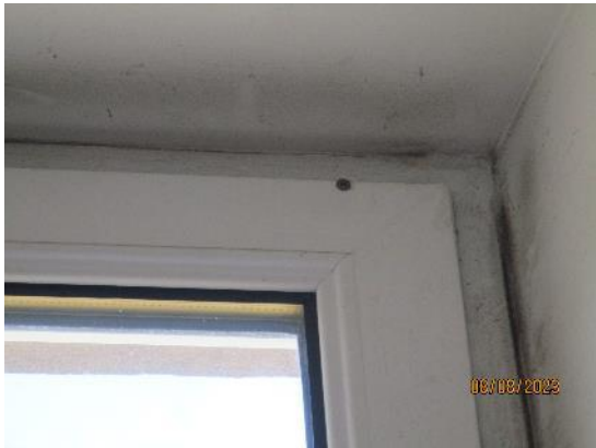
111. Windows screwed shut
