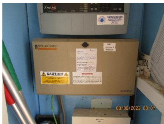
319. Distribution board L+P – nursery.
