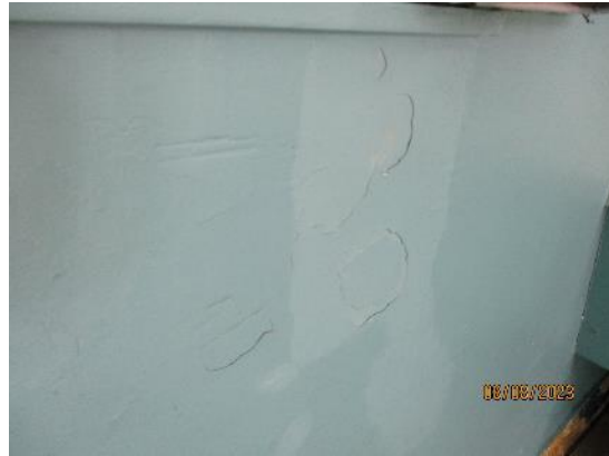
186. Cracked plaster walls
