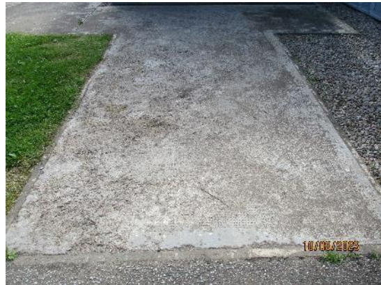
142. Eroded concrete ramp surface
