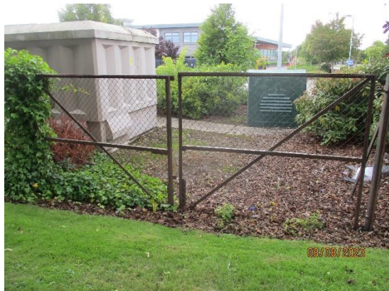
395. Chain link double gate to sub station
