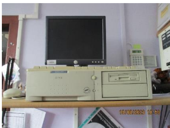
358. CCTV desktop and monitor 1/3 reception.
