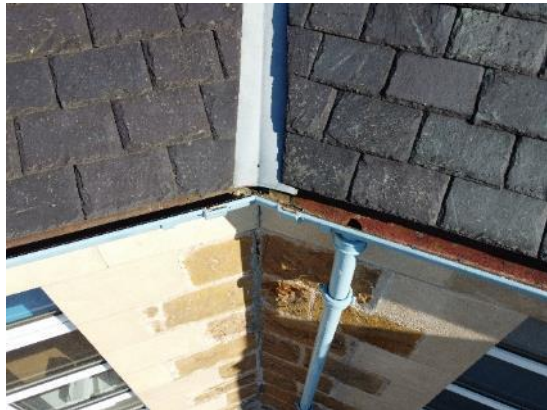
46. Surface corrosion in cast iron gutters
