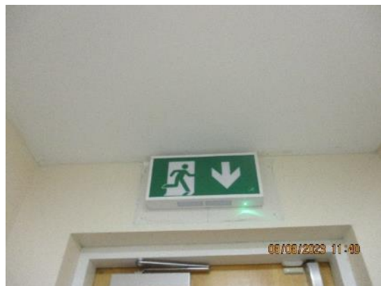
343. Emergency lighting – 2008 extension.
