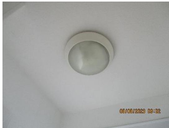
335. Lighting – nursery toilet.
