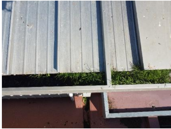
56. Blocked with vegetation
