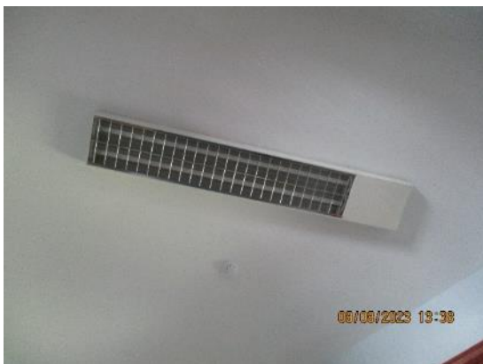
330. Lighting – original school classroom.
