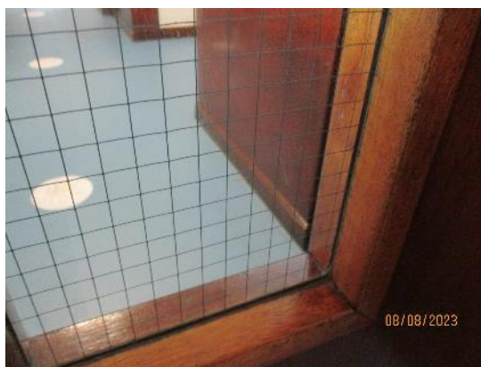
216. Georgian wired glass to internal doors
