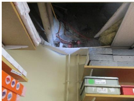
219. Heating pipework block 1 annexe above ceiling.
