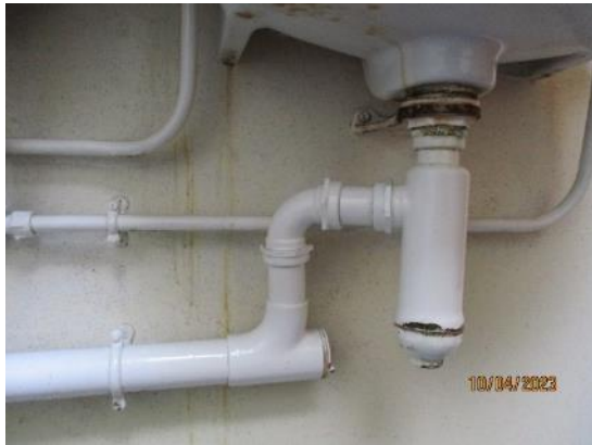
181. Copper waste pipes
