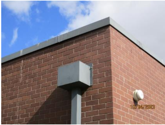
43. Nursery – metal box hopper heads
