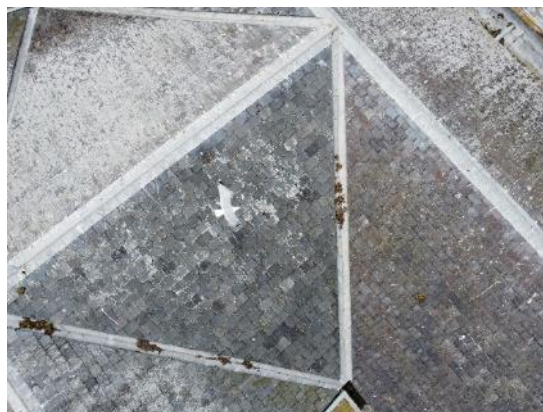
6. Debris in lead valleys
