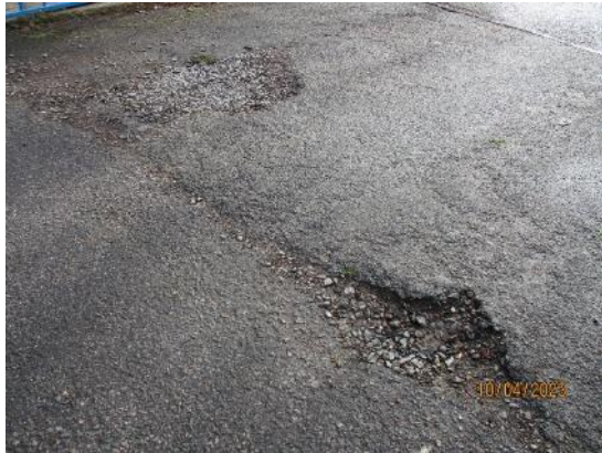
298. Tarmacadam access road - potholes
