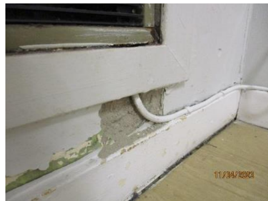
142. Damaged plaster walls
