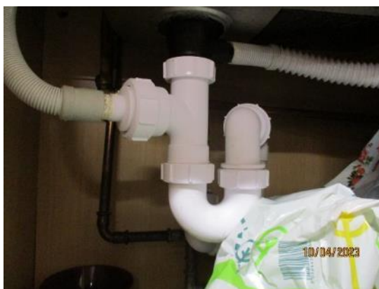
198. UPVC waste pipes
