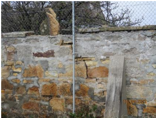
328. Significant damage to stone walls
