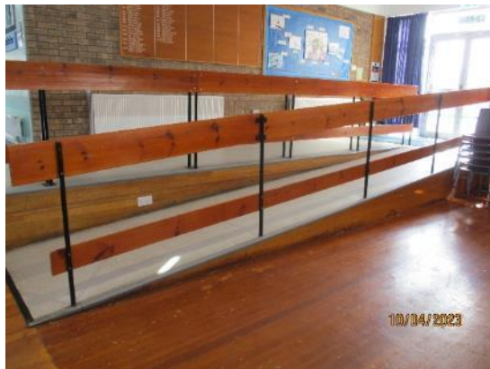
128. Block 2 – Timber handrails
