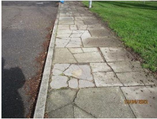
310. Extensively cracked paving slab footpaths
