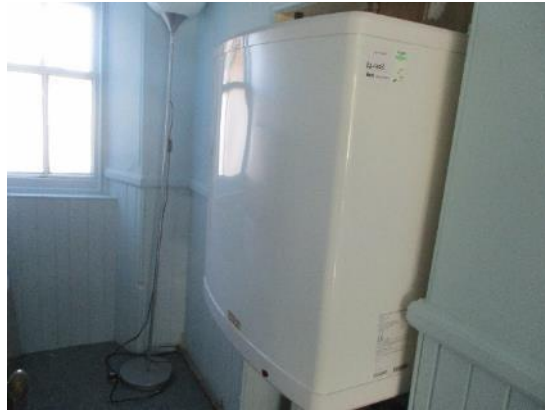
227. Point of use water heater (75L) 2/13 Block 1 annexe.
