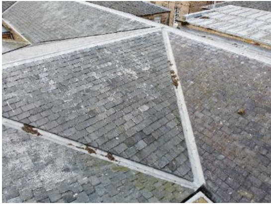
7. Typical slate condition
