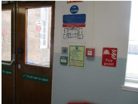
294. Security door devices – push button release/emergency release pad. Block 1 Annexe.
