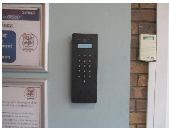
290. Security – door access control unit – block 2. 1/1 corridor.
