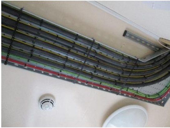
250. Sub mains cabling and containment 1/38 block 2
