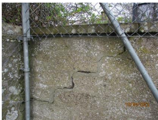
332. Cracked blockwork walls
