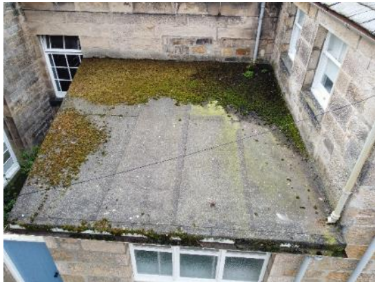
10. Felt roof with extensive moss growth
