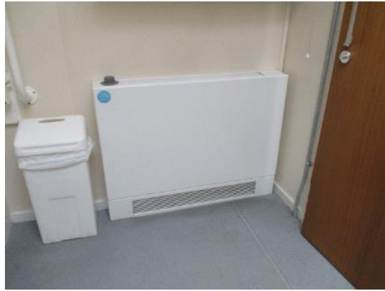
215. Radiator in access toilet 1/23 block 2.
