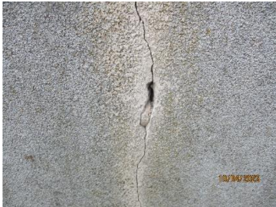
342. Cracked external wall and roughcast
