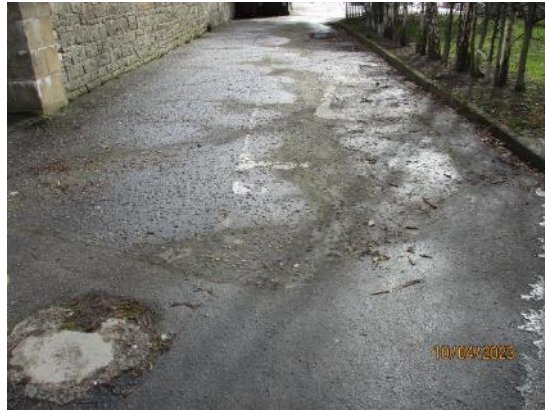
299. Access road subsiding
