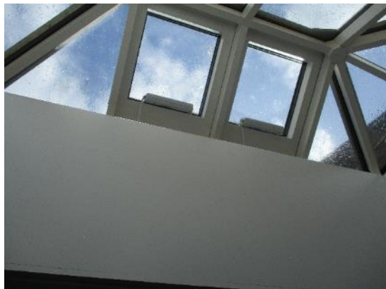
240. Electric windows – 1-21 Block 1 annexe.
