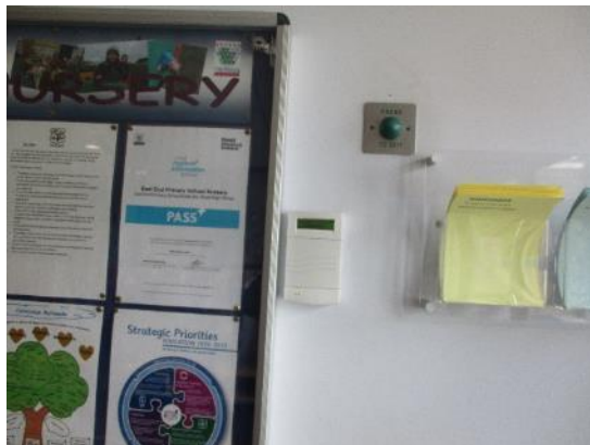
288. Intruder alarm keypad – nursery / access corridor.
