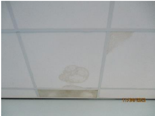
133. Isolated water marking
