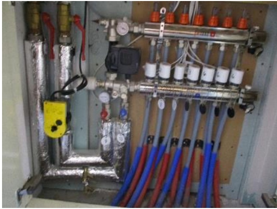
220. Underfloor heating manifold – nursery GO2.
