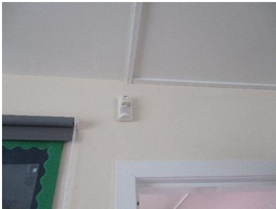
286. Intruder alarm PIR – block 2 typical.
