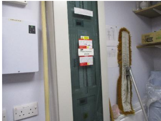
253. Distribution board - Nursery GO1 utility room
