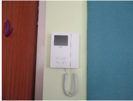
293. Security door access handset – block 1 Annexe.
