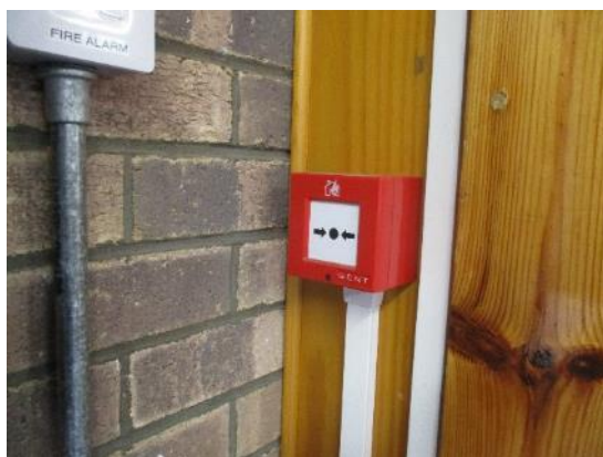
272. Fire alarm system call point block 2 typical.
