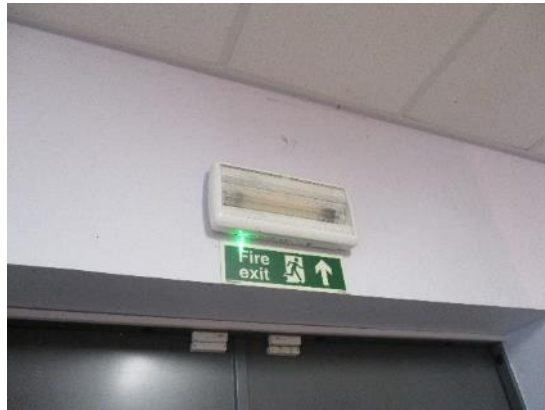
265. Emergency lighting nursery typical.
