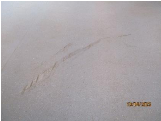
110. Damaged sheet vinyl
