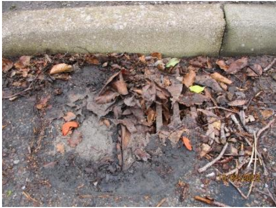
334. Blocked drainage to access road
