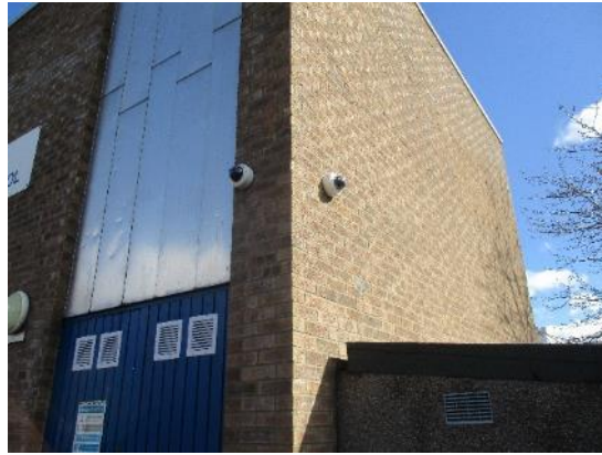
281. CCTV cameras – external block 2 1/33
