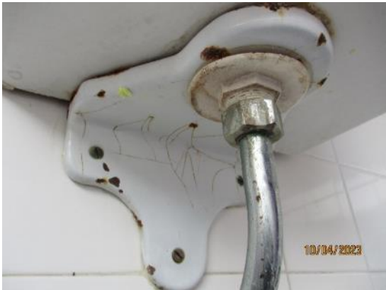
169. Cracked wall brackets
