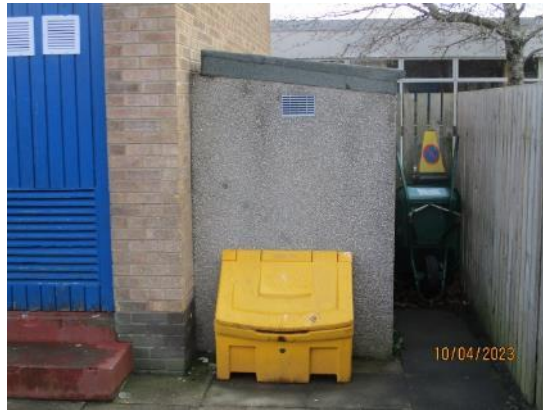
343. Gas meter housing (Block 2)
