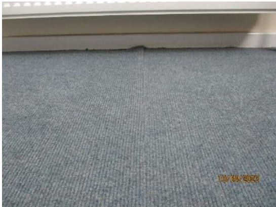
116. Loose carpet edges
