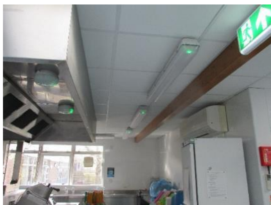
260. Lighting – kitchen 1/3 block 2.
