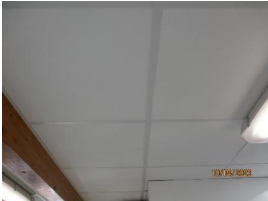
131. Suspended ceiling tiles
