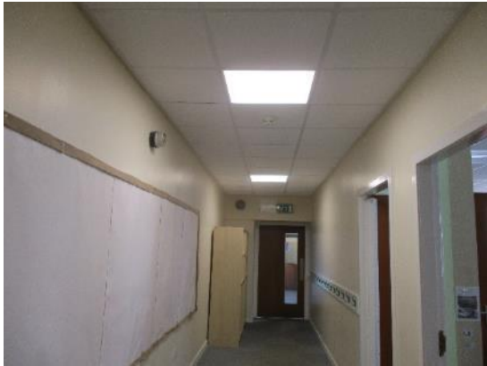
268. Lighting corridor block 1 typical
