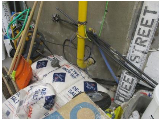
235. Gas pipework 1/33 block 2.
