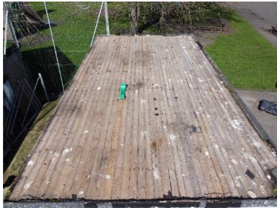
22. Felt stripped exposing timber boards
