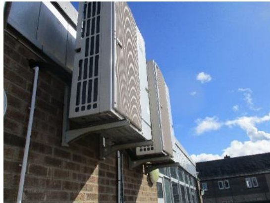
247. Air conditioning outdoor units classes 1/13 + 1/15.
