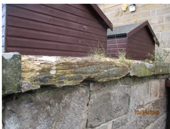
326. Eroded coping stones
