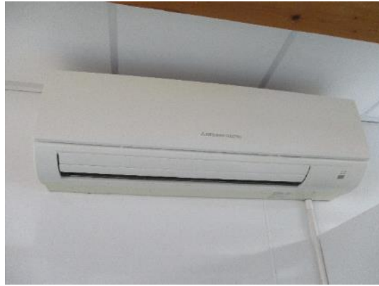
245. Air conditioning indoor unit - kitchen 1/3 block 2.
