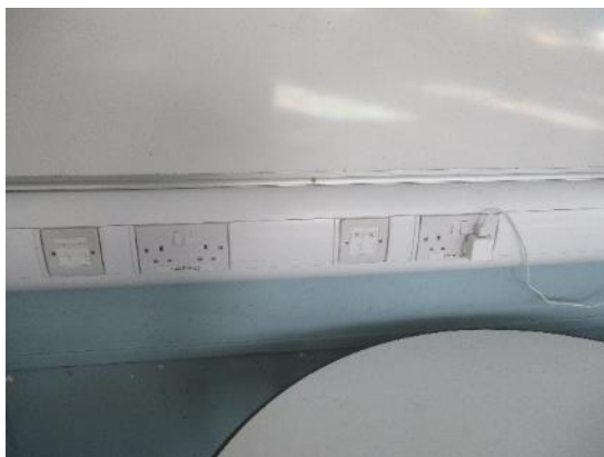
255. Sockets and switches typical block 1
