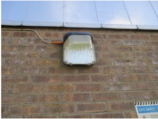
262. External lighting block 2 typical.
