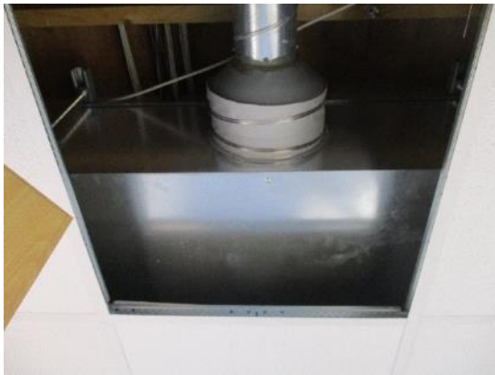
238. Ventilation unit – Nursery above GO3 access WC.
