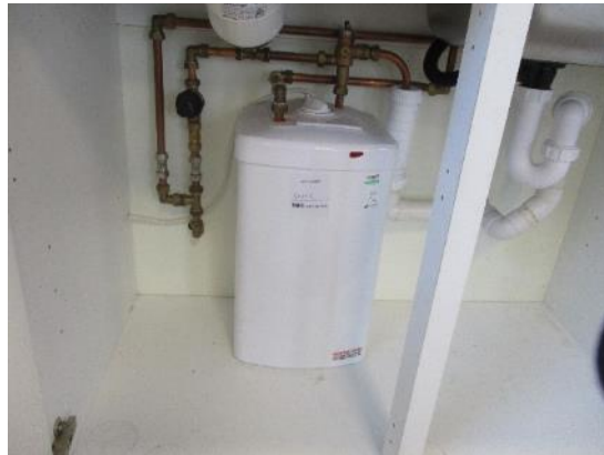
229. Point of use water heater block 1 annexe typical.
