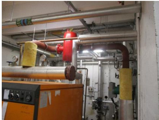
211. Heating pipework 1/33 block 2.
