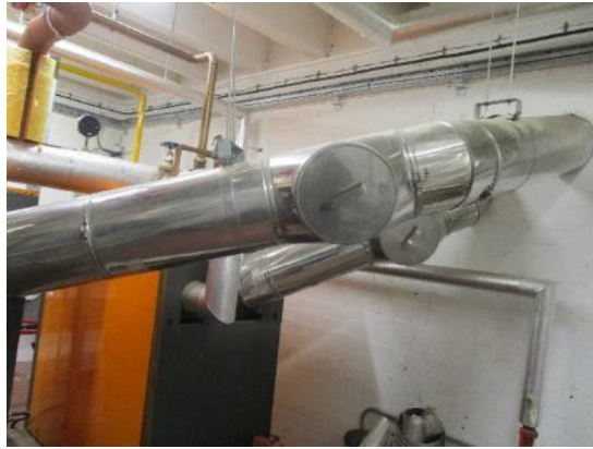
209. Boiler flues into brick chimney. 1/33 block 2.
