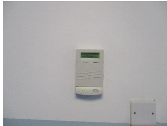
287. Intruder alarm keypad – block 1 annexe.
