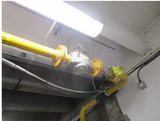
234. Gas supply solenoid valve 1/33 block 2.
