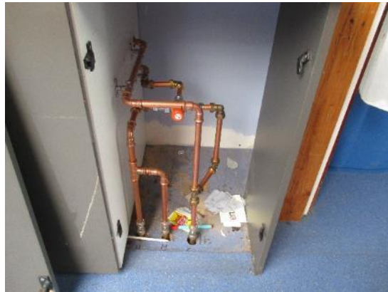
223. Hot water pipework – block 2 typical.
