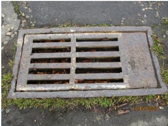
336. Blocked drainage to playground
