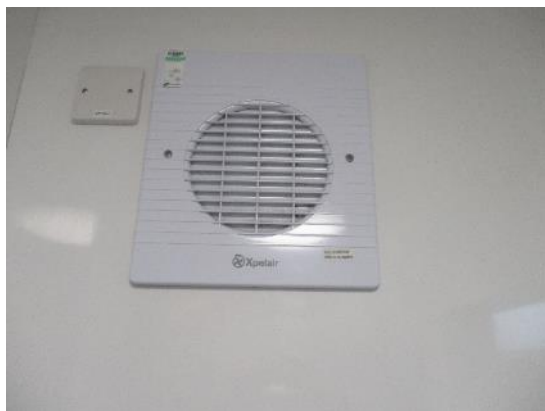
236. Extract fan – kitchen store block 2. 1/2
