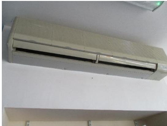
246. Air conditioning indoor unit class 1/13 (P5)
