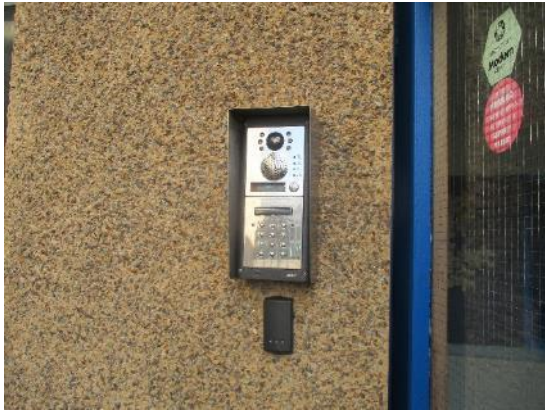
292. Security door access control block 1 Annexe.
