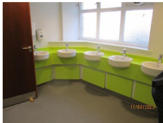
190. Vanity base units (Block 1)
