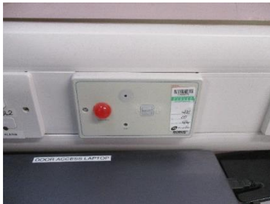
276. Disabled toilet alarm system alert panel block 2 1/25
