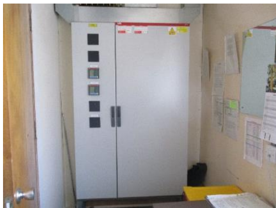
248. Main distribution board block 2 – room 1-38
