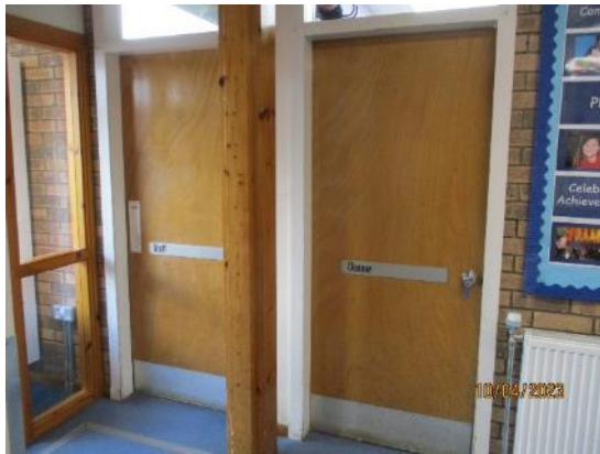
155. Block 2 – Varnished timber doors
