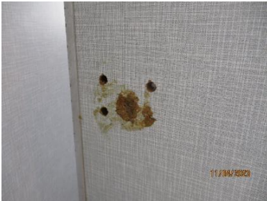
187. Damaged cubicle partitions
