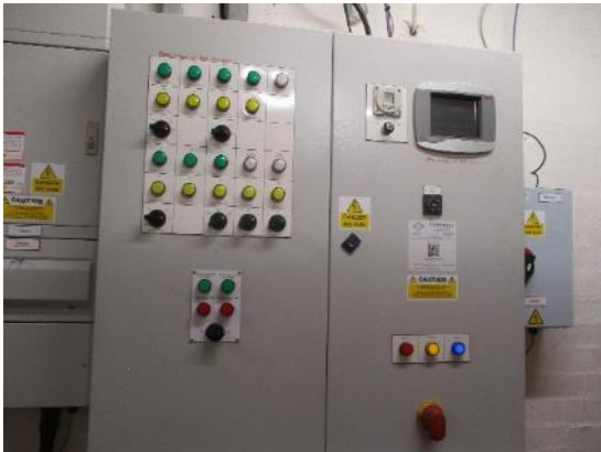
210. Heating control panel 1/33 block 2.
