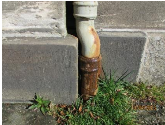
38. Cracked, leaking, corroded cast iron
