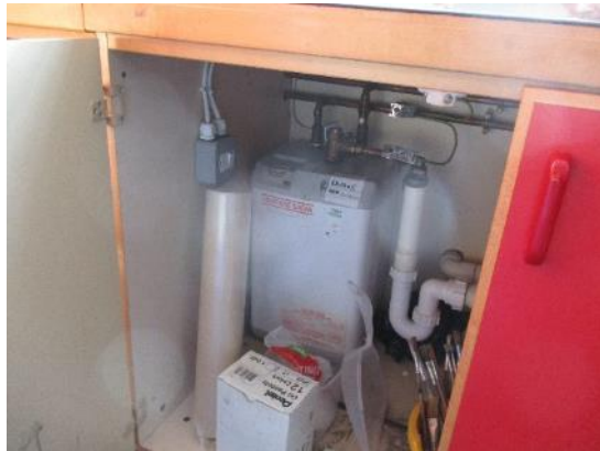
228. Point of use undersink water heater – block 1 annexe. Room 1/19
