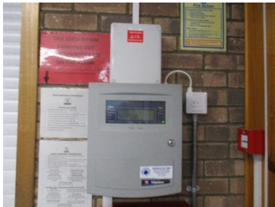
270. Fire alarm control panel – block 2. 1/1
