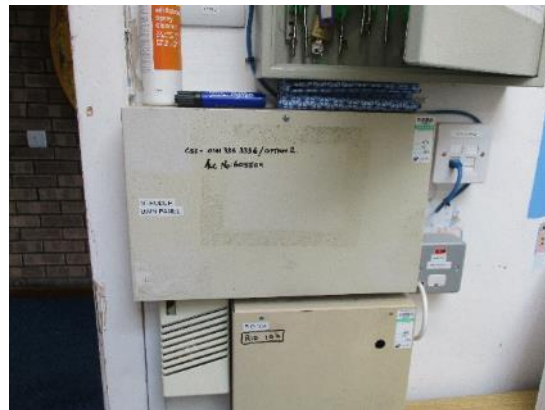
289. Intruder alarm panel – block 2.
