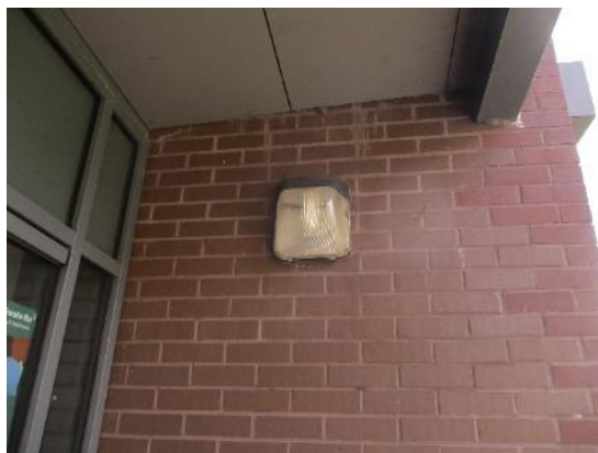
266. External lighting nursery typical.
