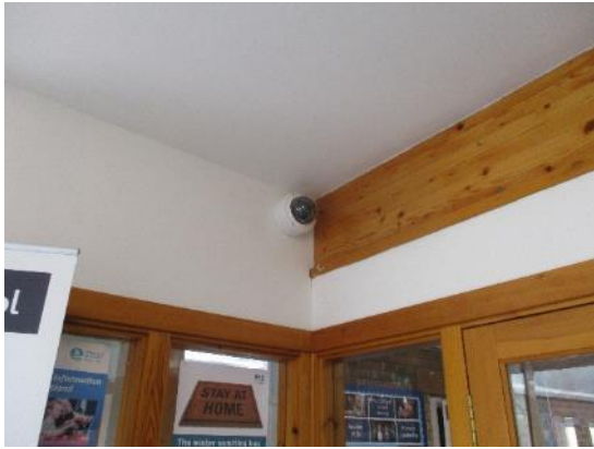
280. CCTV camera block 2 main entrance.
