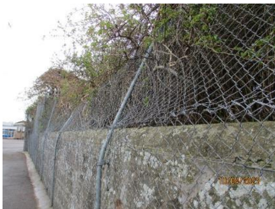
315. Damage to chain link fencing
