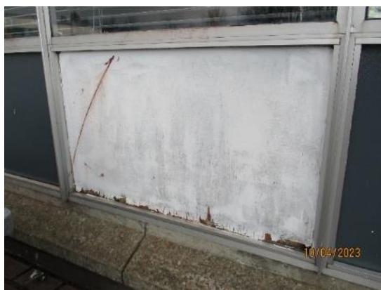
78. Defective panel below windows
