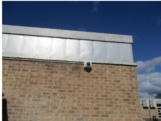
283. CCTV camera – nursery external.
