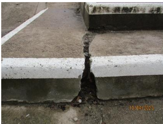
100. Broken concrete steps
