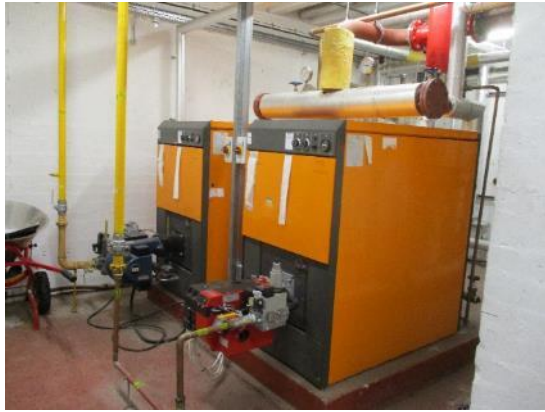
208. Natural gas boilers 1/33 block 2.
