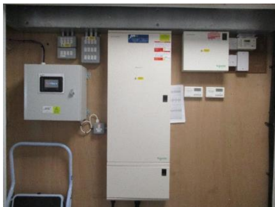
254. Distribution boards - electric cupboard 1/14 block 1
