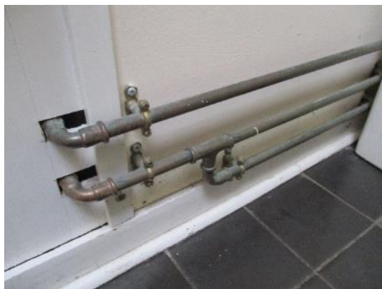
230. Cold water pipework – block 2 1/32 typical.
