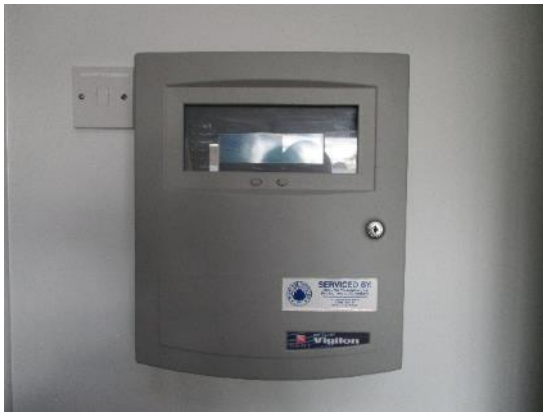
274. Fire alarm control panel block 1 reception.
