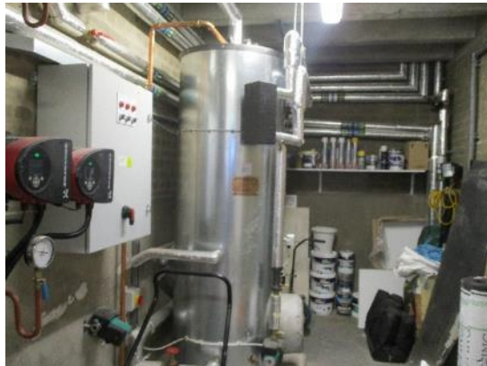
222. Hot water calorifier 1/33a – Block 2.
