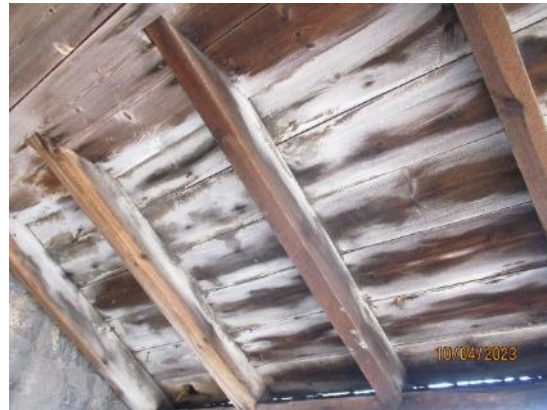
140. Evidence of rainwater penetration
