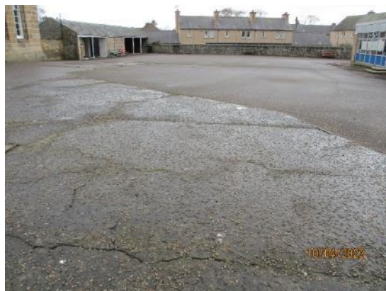
303. Tarmacadam playground cracking
