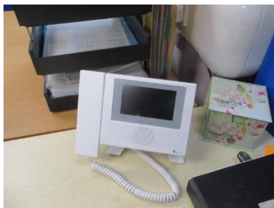
291. Door entry user control handset and monitor – block 2 reception office 1/25.
