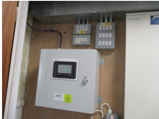
217. BMS Heating control panel block 1 annexe.
