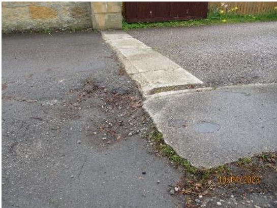
300. Access road - uneven
