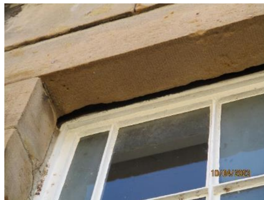
73. Gaps around windows
