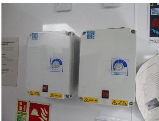
243. Extract canopy fan controls. 1/3 kitchen block 2.
