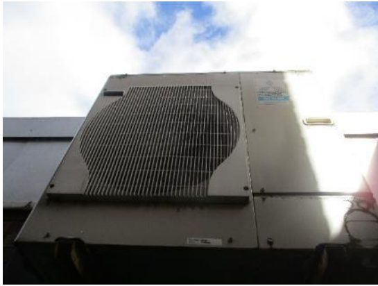
244. Air conditioning outdoor unit - kitchen 1/3 block 2.
