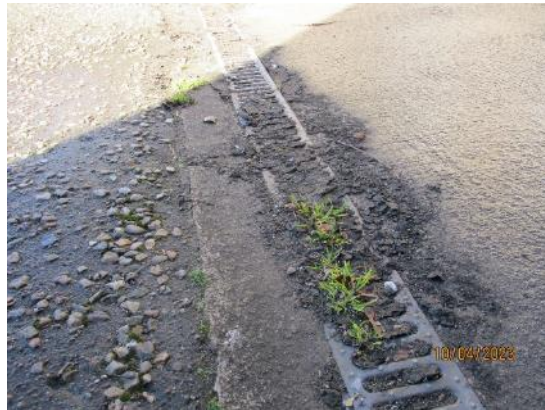
337. Blocked channel drain to Block 1
