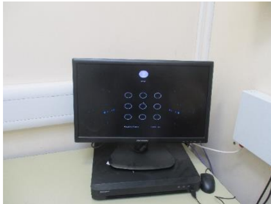
282. CCTV monitor and recorder block 2 1/24
