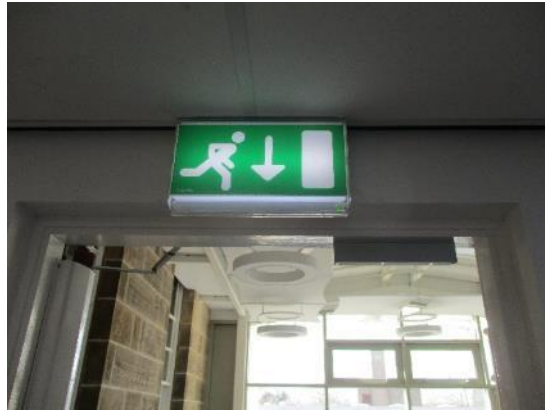
269. Emergency lighting dedicated exit – block 1.
