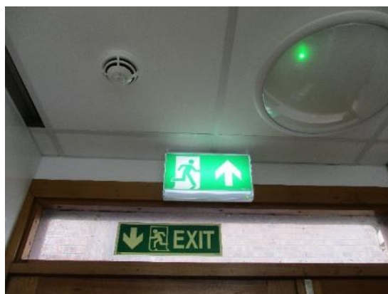
261. Emergency lighting – block 2 typical.
