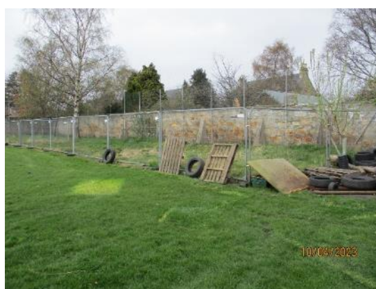
327. Damage to perimeter wall
