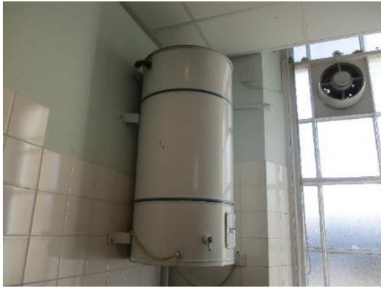
226. Hot water calorifier girls 1/2 block 1 annexe.
