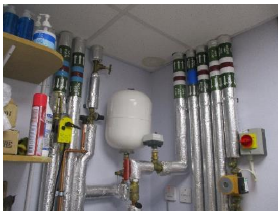
225. Hot water pipework – nursery GO2.
