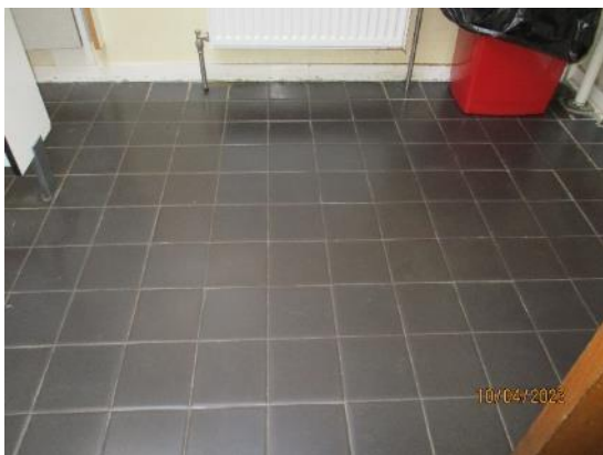
118. Quarry tiles in toilets
