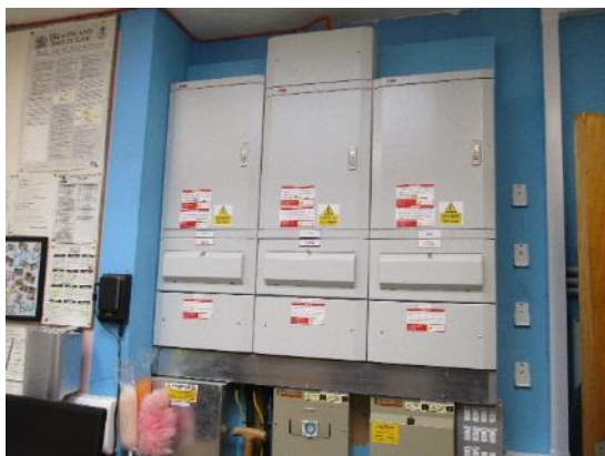
249. DBs – Janitors room block 2
