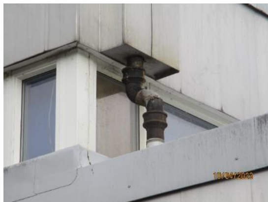
42. Poor condition downpipes
