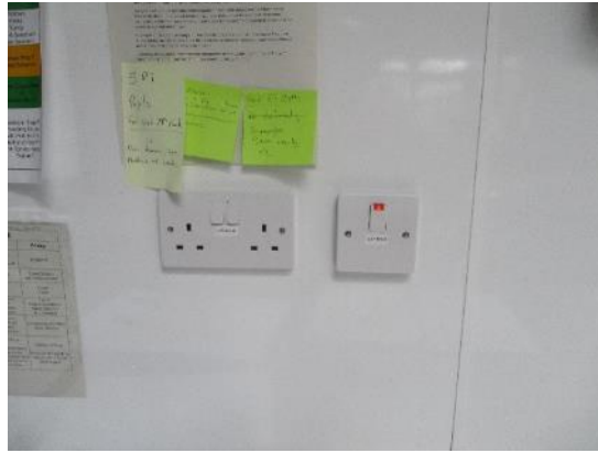
251. Sockets and switches kitchen 1/3 block 2
