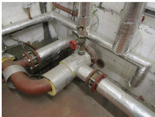
213. Heating pipework 1/33 block 2.
