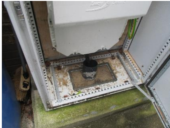
252. Incoming power supply outside kitchen 1/3 block 2
