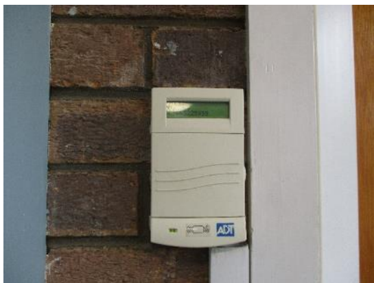
285. Intruder alarm keypad block 2. 1/1 corridor.
