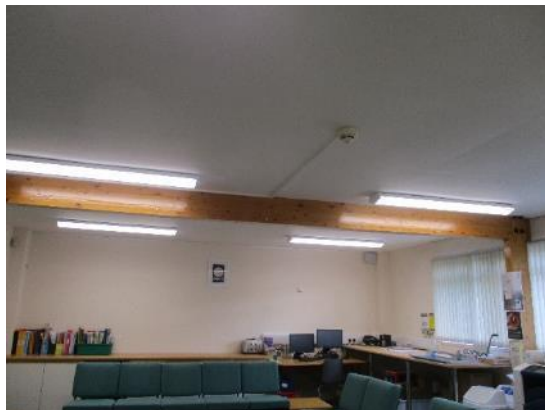
258. Lighting – staffroom block 2. 1/30
