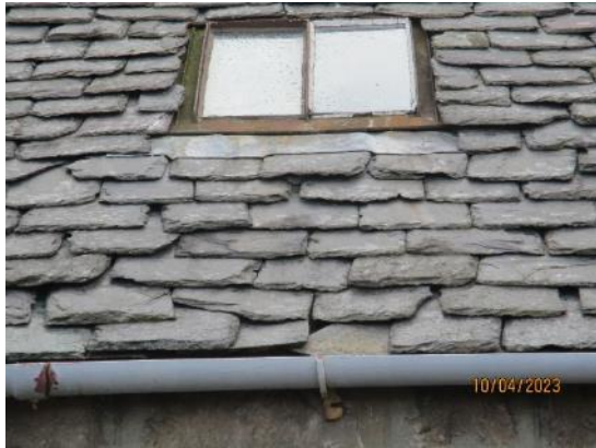
13. External shelter – poor slate
