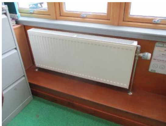
182. Radiator – typical throughout.
