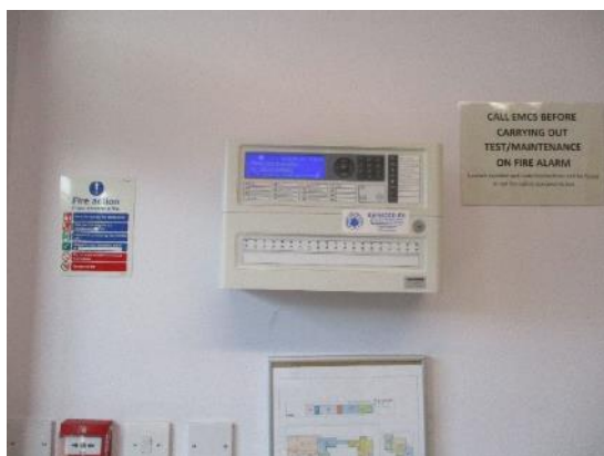
214. Fire alarm control panel – hub building.
