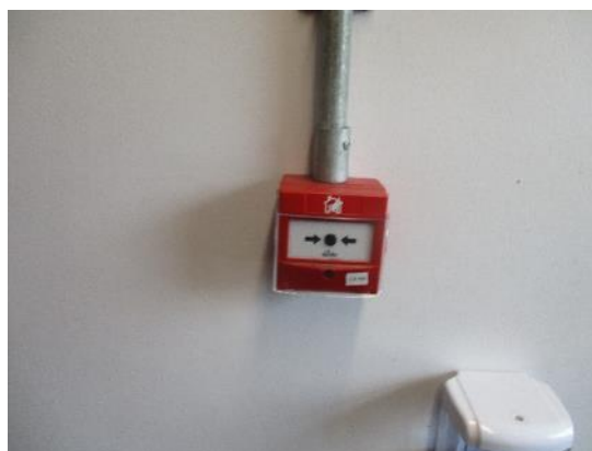
215. Fire alarm call point typical throughout.
