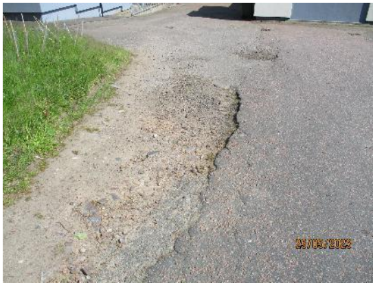
238. Access road to Kitchen breaking up
