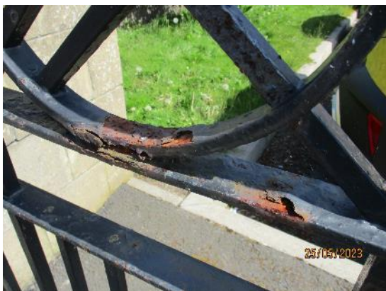
260. Peeling paint and surface corrosion
