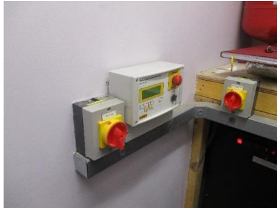
197. Gas safety control panel – hub plant room.
