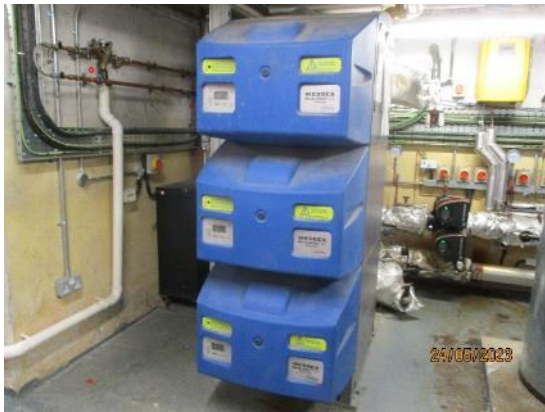
178. Main school and modular building boilers.
