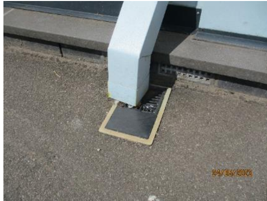
38. Downpipes miss-aligned with drainage
