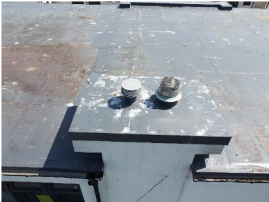
39. Boiler flue and terminals
