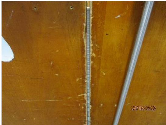
128. Gaps with damage to edges
