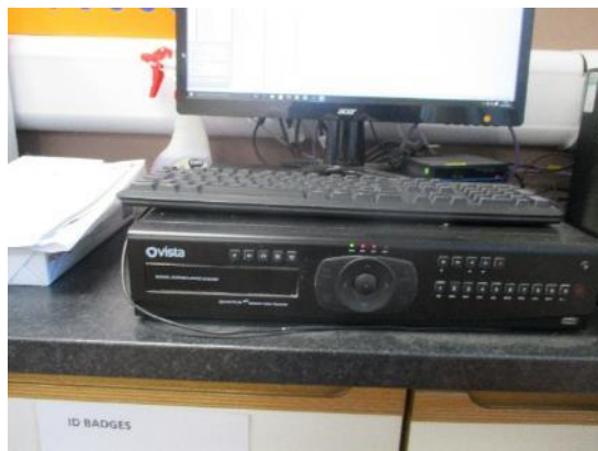
231. CCTV system recorder and monitor main school.
