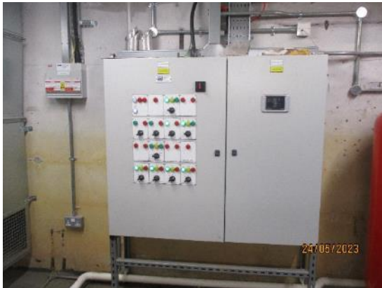
180. Control panel main school boilerhouse.
