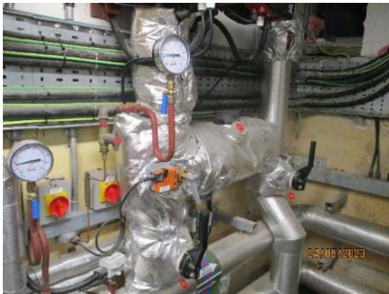
184. Heating pipework main school boiler house.
