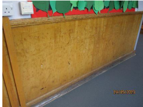
115. Minor surface damage
