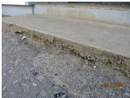
78. Eroded concrete steps
