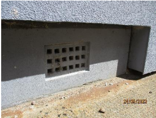
43. Primary school underfloor ventilation
