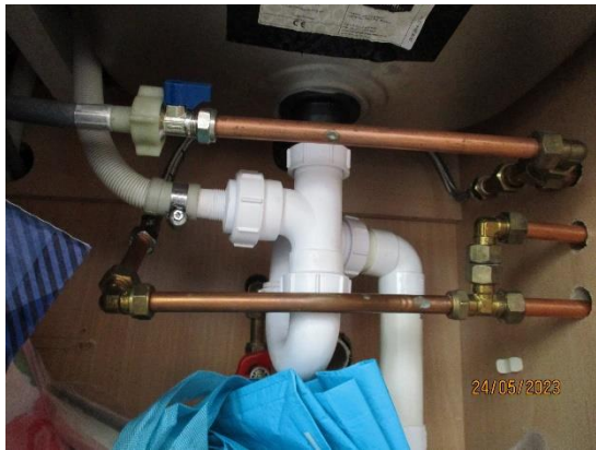
162. PVC waste pipes
