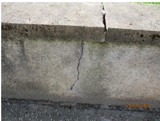
272. Cracks to brick walls
