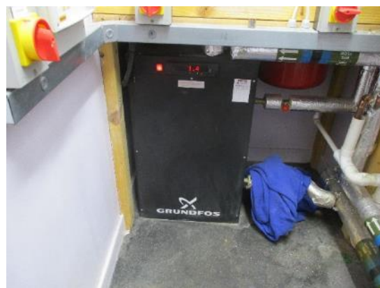
189. Pressurisation unity – hub building.
