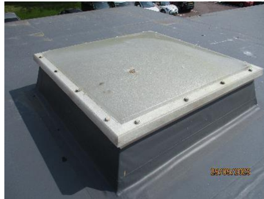
16. GRP Rooflights to Primary School
