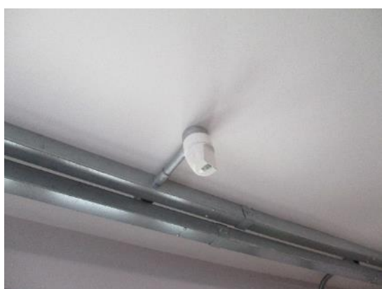
218. Lighting – PIR control main school typical.
