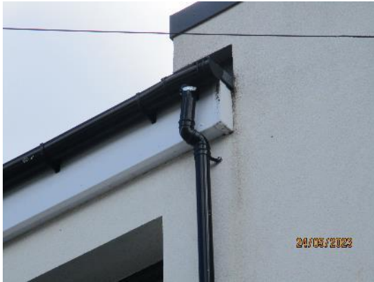
25. UPVC downpipes (isolated defects)
