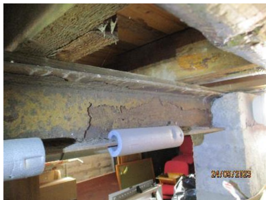
84. Corroded steel beams
