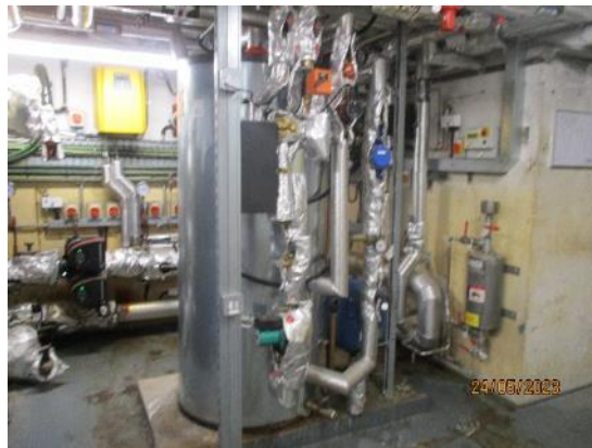
187. Hot water calorifier – main school boiler house.
