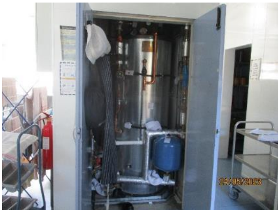
186. Hot water calorifier – main school kitchen.
