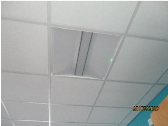
220. Lighting (with emergency self-contained) modular nursery building corridor.
