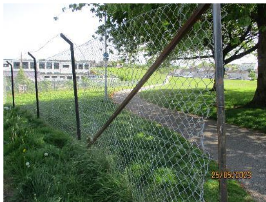
255. Loose chain link fencing
