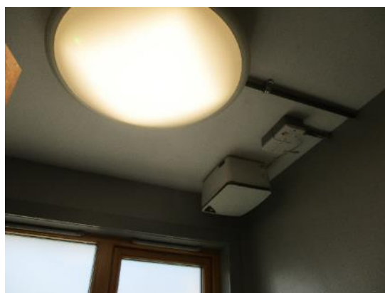
217. Lighting – toilets and stores generally. Main school.
