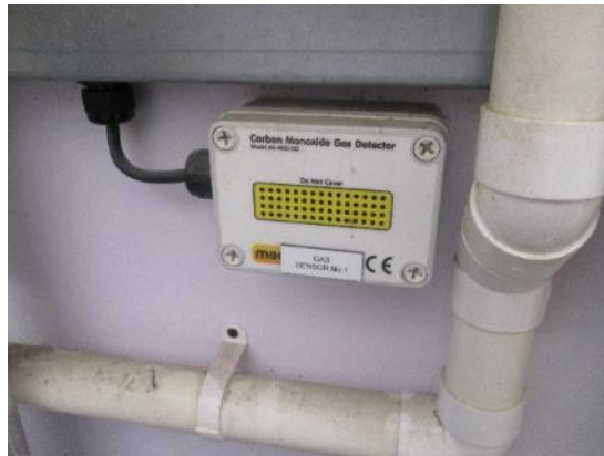
185. Carbon monoxide detector hub boiler house.
