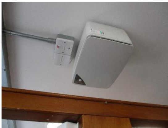
194. Extract fan – typical throughout all 3 buildings.
