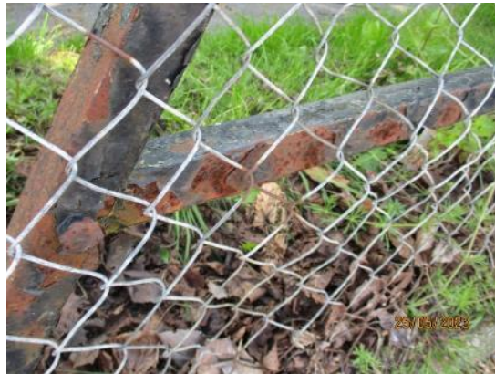
76. Surface corrosion to fence framework
