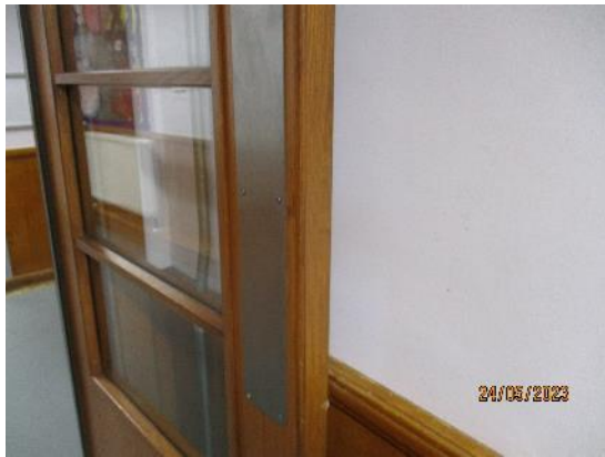
126. Not all are fire doors
