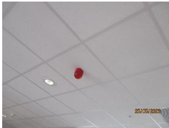
211. Fire alarm strobe – modular nursery building.
