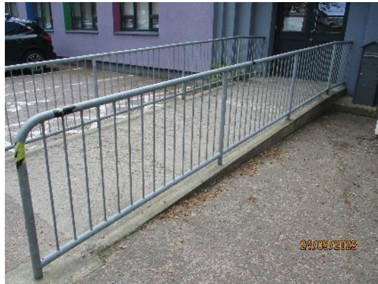
82. Galvanised guard rails to ramps
