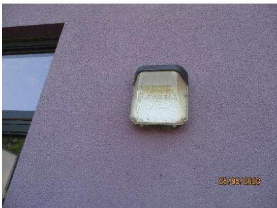
236. External lighting modular nursery building.
