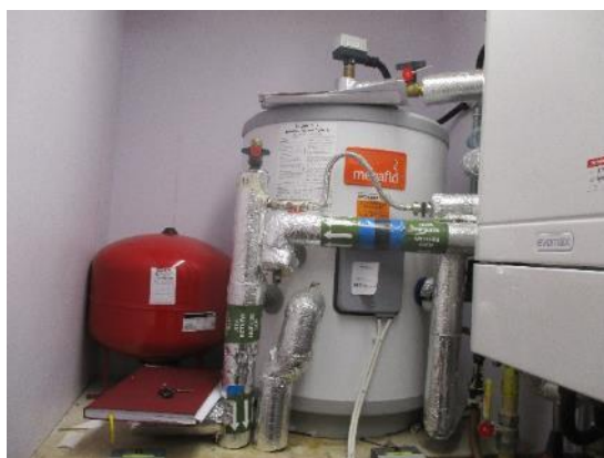
188. Hot water storage tank – hub building.
