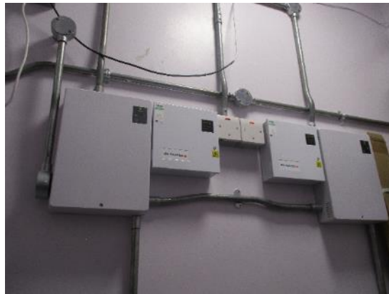
227. Door security control panels main school.
