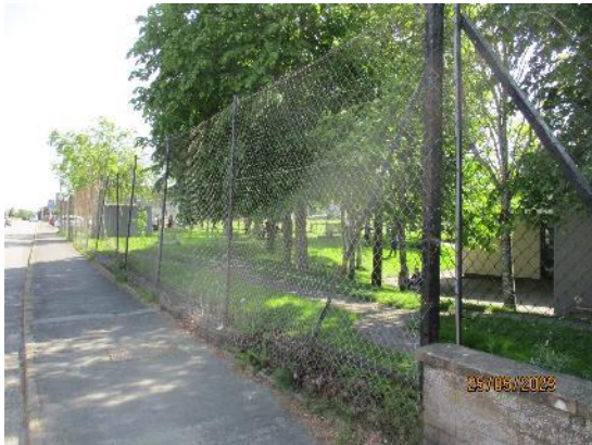
252. Chain link fence leaning
