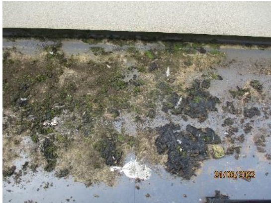
13. Bird droppings and vegetation
