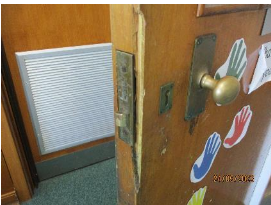
124. Damage to door edges
