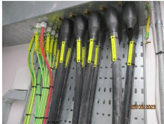
205. Sub mains cabling – main school.
