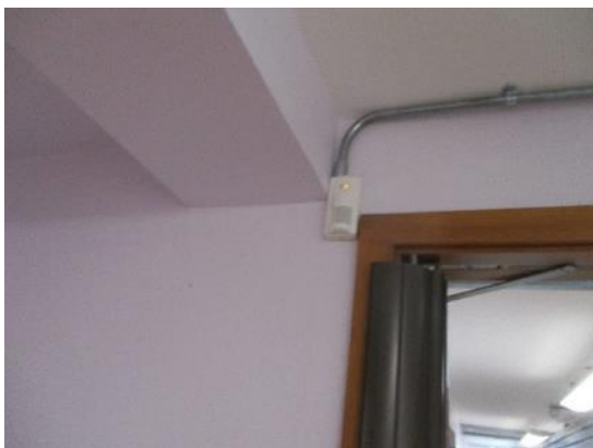
224. Intruder alarm PIR sensor – main school.
