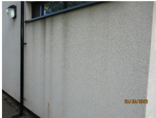
74. Staining to external insulation
