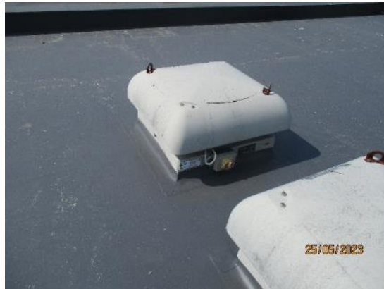
199. Extract fan terminals – main school kitchen on roof.
