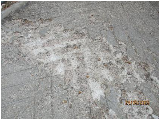
81. Surface breaking up
