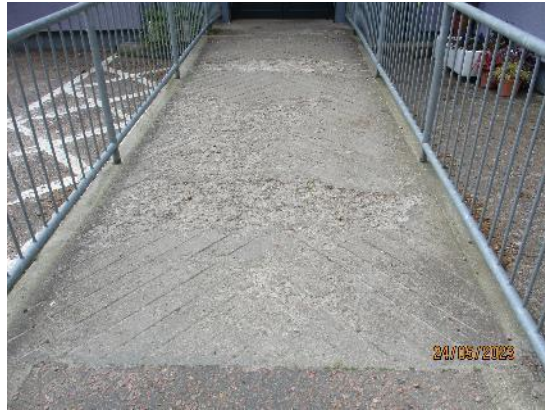
80. Eroded concrete entrance ramp
