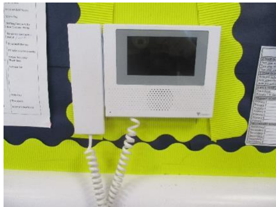
229. Security door system user handset and monitor screen main school.
