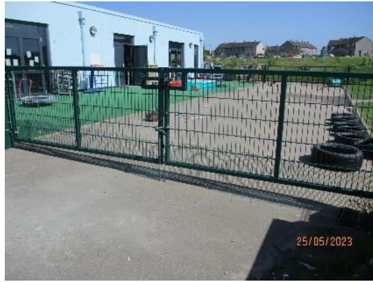
263. Security mesh vehicle gates
