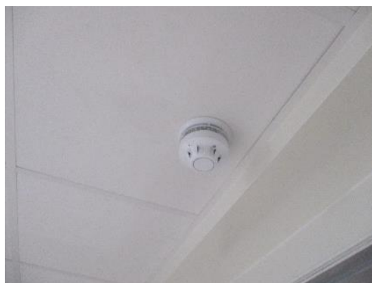
213. Smoke detector – typical throughout 3 buildings.
