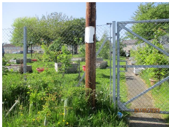
285. Timber utility pole
