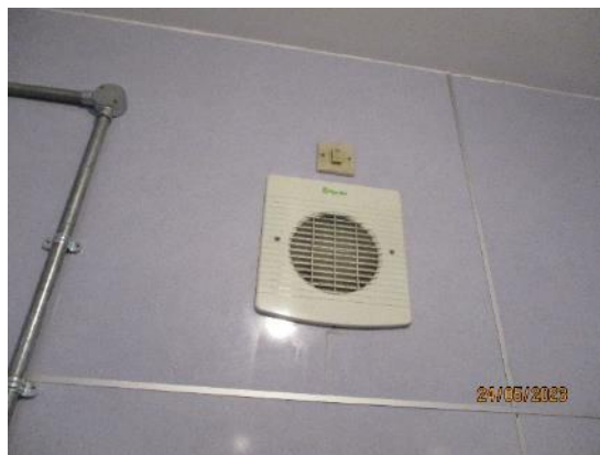
195. Extract fan – kitchen store main school.
