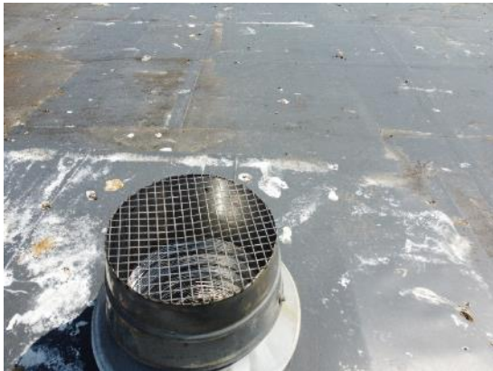
234. Boiler flue roof termination – main school.
