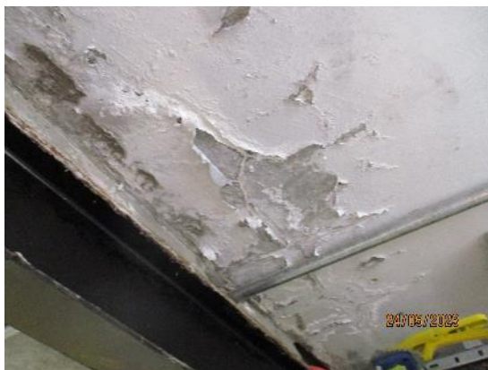
107. Concrete ceiling, peeling paint
