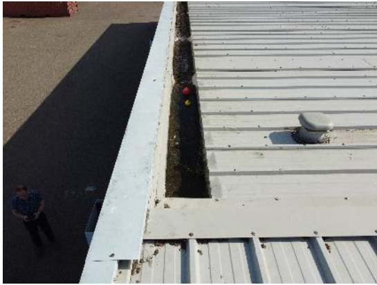
31. Box gutters with standing water
