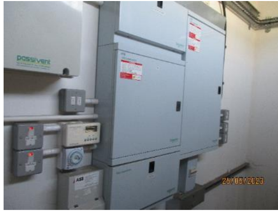
203. Distribution boards – modular nursery building.
