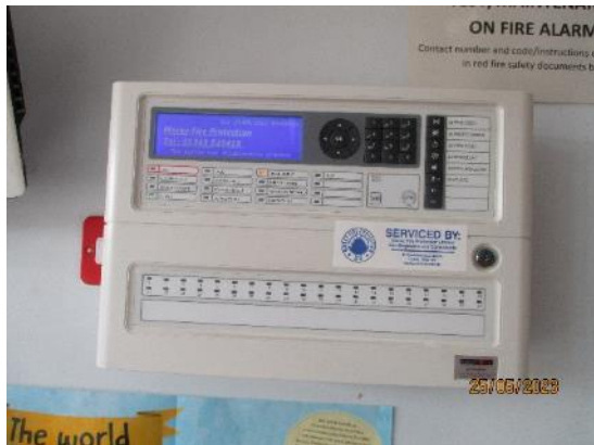
210. Fire alarm control panel – modular nursery building
