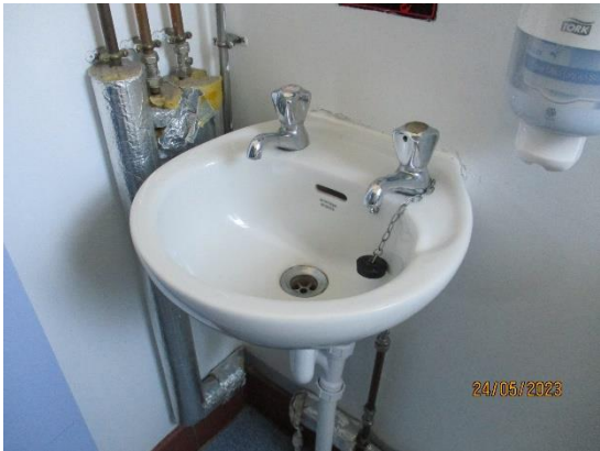
146. Wall hung wash hand basin
