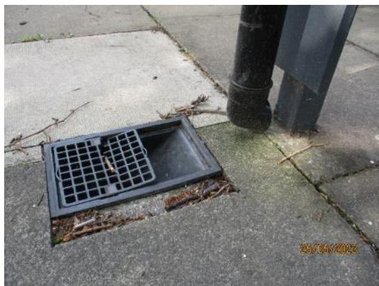
35. Downpipes not discharging to drainage
