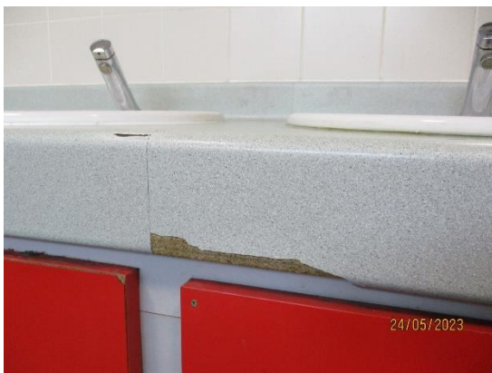
154. Isolated surface damage
