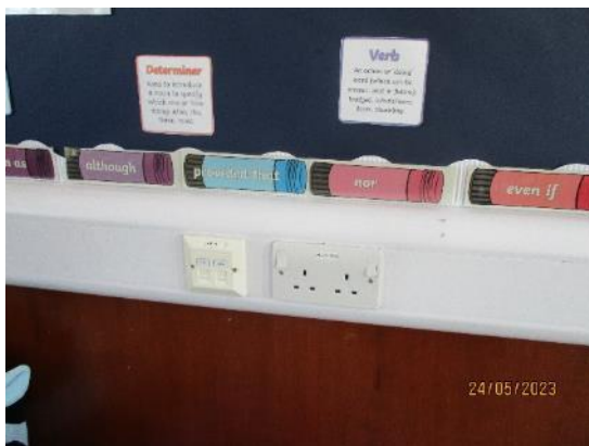
207. Wiring accessories – main school.
