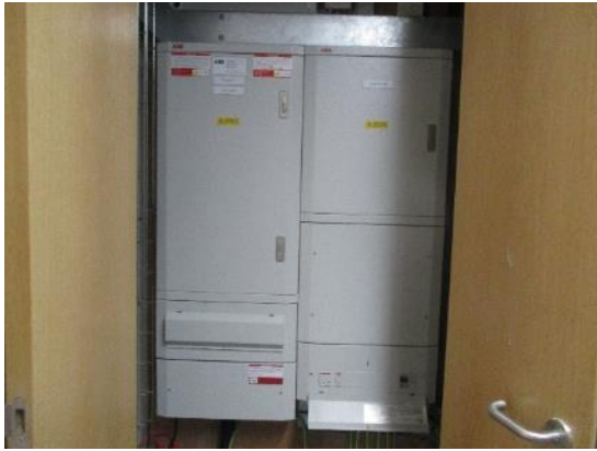
202. Distribution boards – Hub building.
