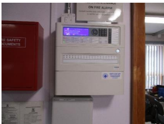
212. Fire alarm control panel main school.
