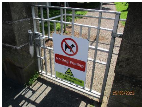
261. Metal bar pedestrian gates
