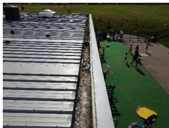
30. Metal roof box gutters, partially blocked
