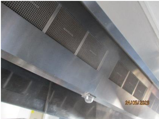
198. Extract canopy – main school kitchen.
