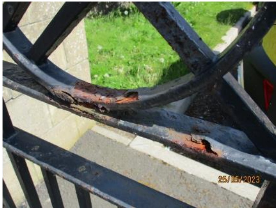
75. Surface corrosion to metal gates
