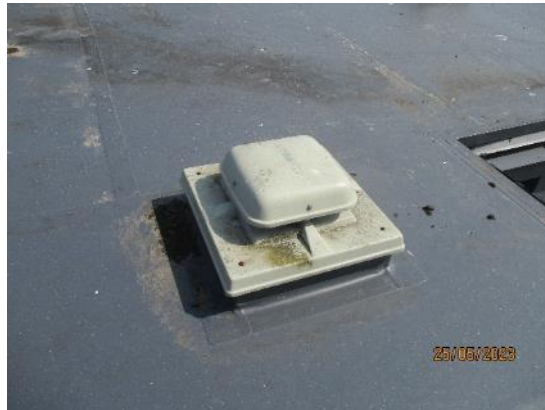
193. Extract fan roof unit – main school external.
