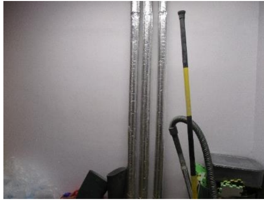
191. Pipework – hot and cold typical throughout.
