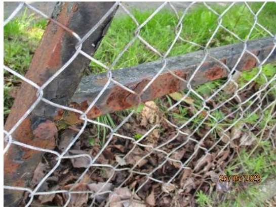
253. Corroded steel frame
