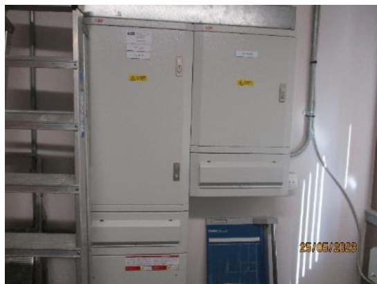
201. Distribution board LP1 main school.
