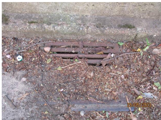
276. Blocked surface water drainage
