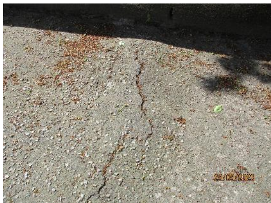
246. Cracking due to tree roots
