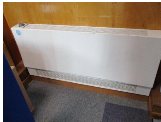
183. LST Radiator typical throughout.
