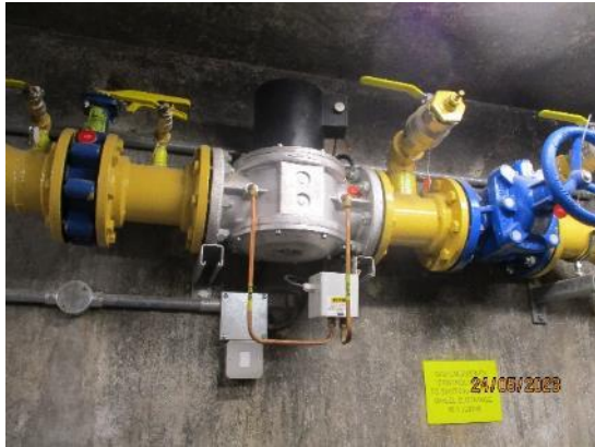
196. Gas supply pipework and solenoid control valve – main school plant room.
