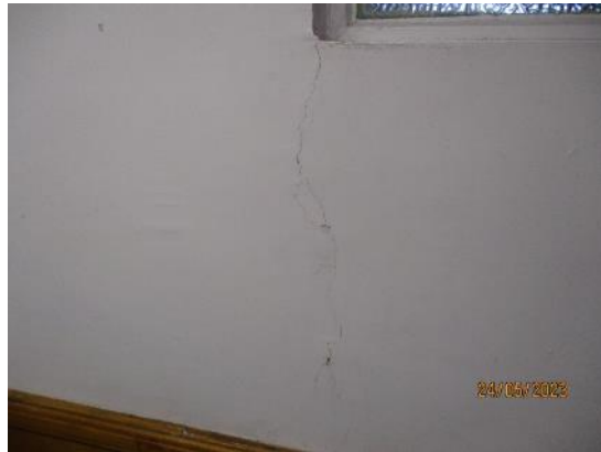
111. Plastered walls (isolated hairline cracking)
