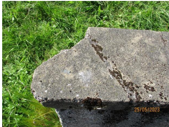
271. Broken coping stones
