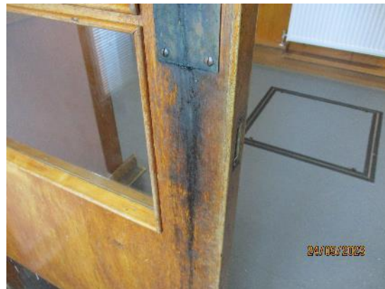
123. Damage to the surface of doors
