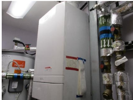
179. Hub building gas condensing boiler.
