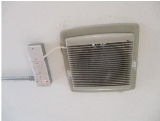
192. Extract fan main school roof mounted. Girls toilets.
