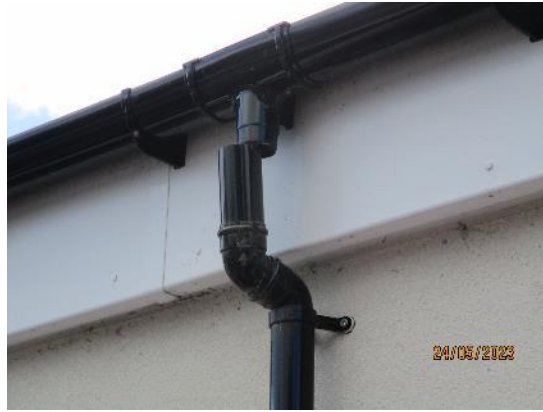
32. UPVC downpipes (isolated defects)
