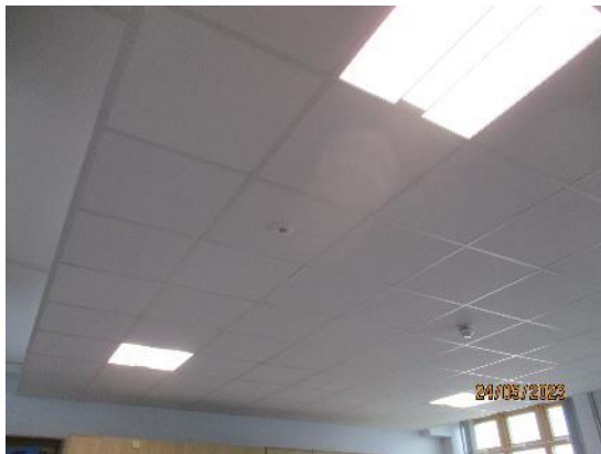
105. Primary school suspended ceiling tiles
