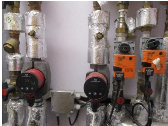
181. Heating pipework and pumps hub building boiler house.
