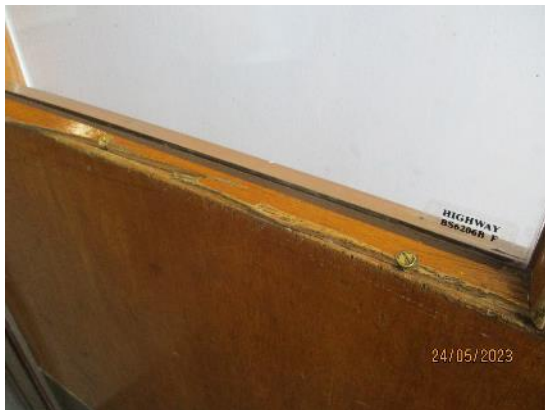
122. Broken glazing beads
