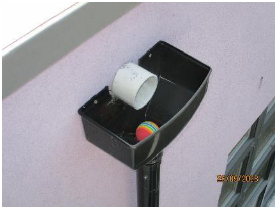
33. Hopper heads with blockages
