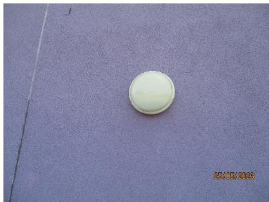
237. External lighting modular nursery building.
