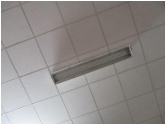
222. Lighting – main school hall.
