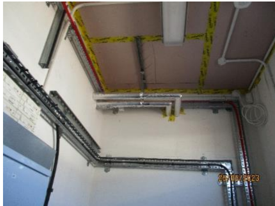
204. Sub mains cabling – modular nursery plant room.
