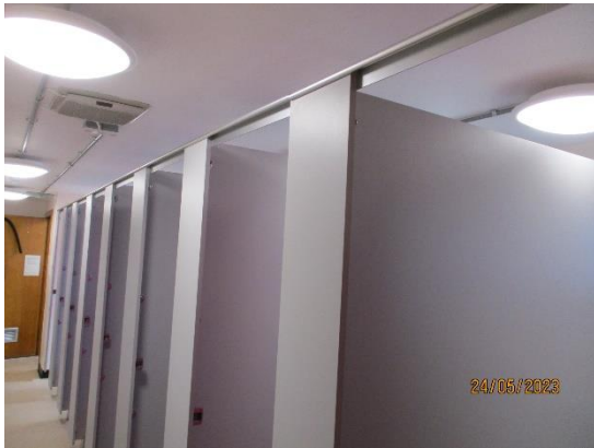
152. Composite panel cubicle partitions
