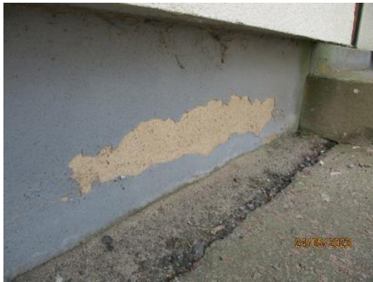
73. Peeling paint to base course
