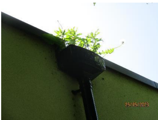
29. Hopper heads, partially blocked with vegetation
