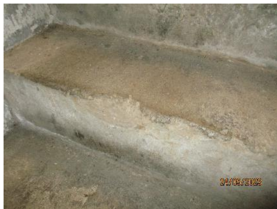
102. Damaged stair nosings
