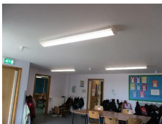
219. Lighting – Hub classroom.
