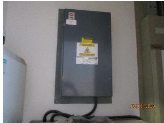
160. DB – emergency lighting 1-11a
