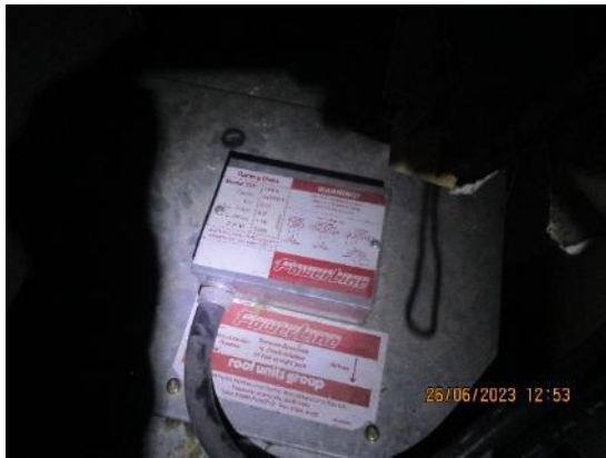
153. Air handling unit attic space.
