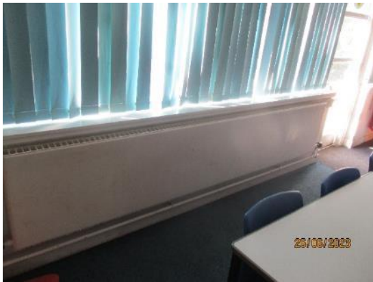
141. Radiator heating system typical 1/11
