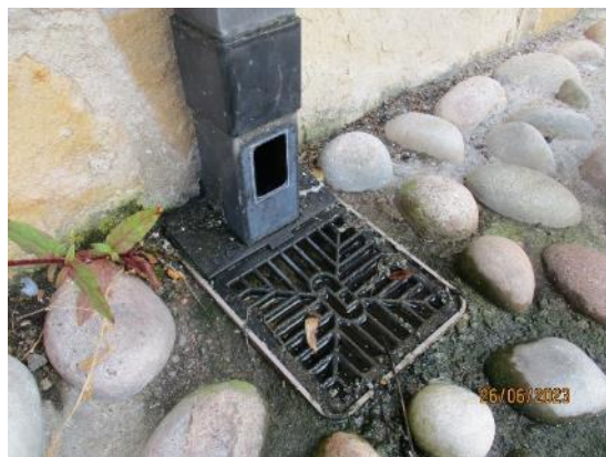
30. Below ground drainage blocked
