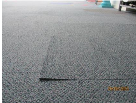
61. Carpet tiles lifting
