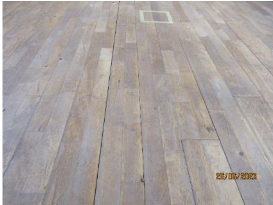
66. Timber boards worn
