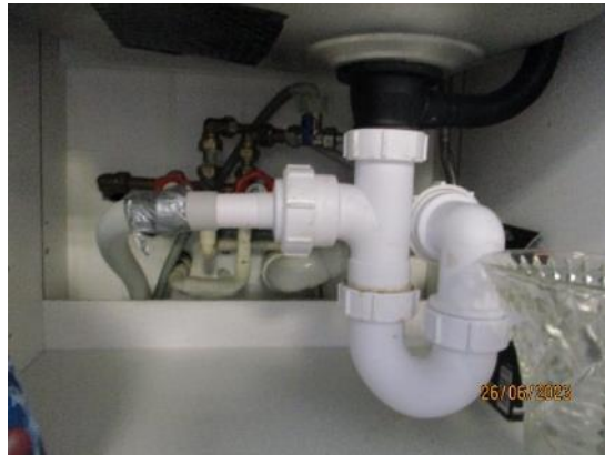
119. PVC waste pipes
