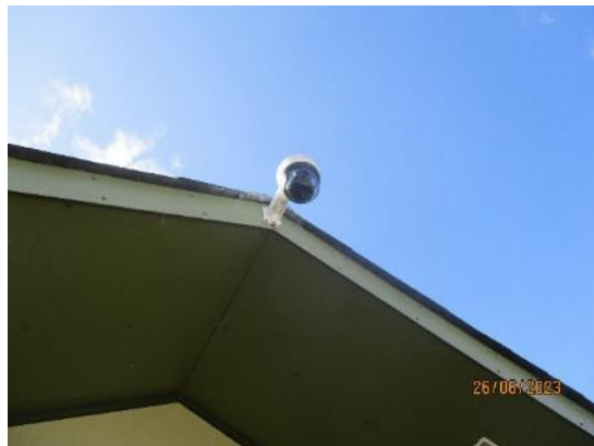
186. CCTV camera south end entrance.
