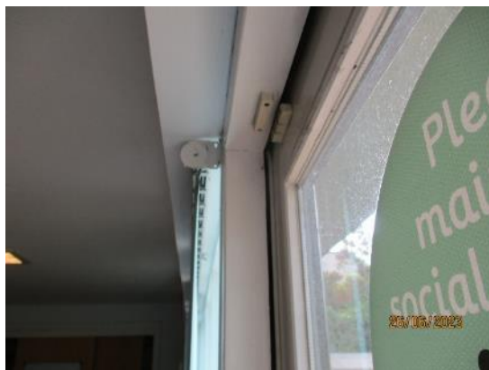
35. Doors twisting, poor fit in frame
