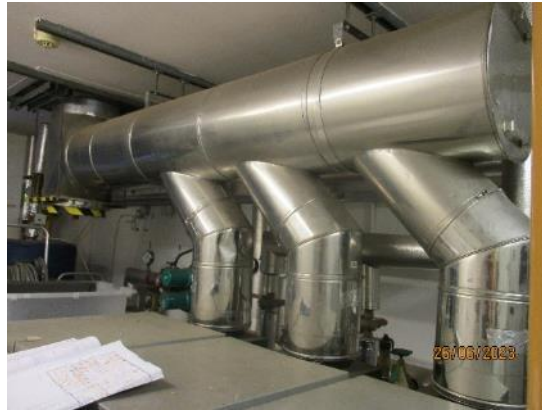
136. Flue system – boilers
