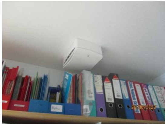
150. Extract fan – cupboard next to kitchen.
