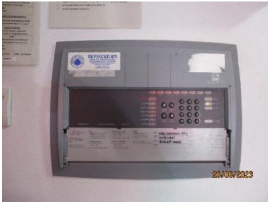
179. Fire alarm system control panel.
