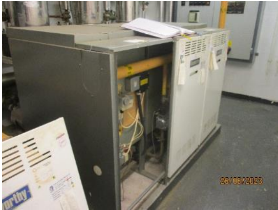
135. Gas boilers – plant room
