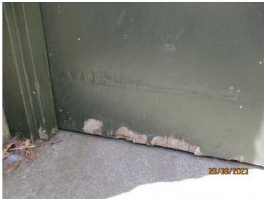
37. Damage to face of doors
