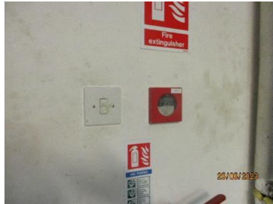
180. Fire alarm system call point typical.
