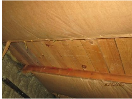
26. Insulation roll collapsed from sarking
