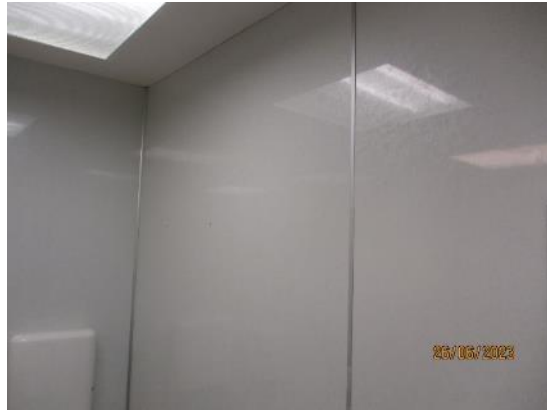
83. Wetwall to boys' toilets
