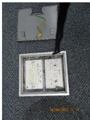
163. Floor socket compartment boxes 1-11
