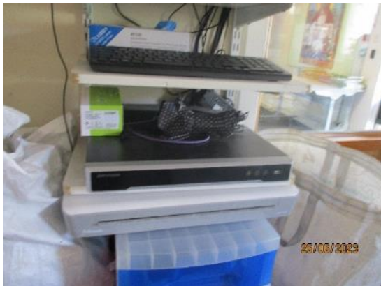
185. CCTV recorder and processor 1/24 office.
