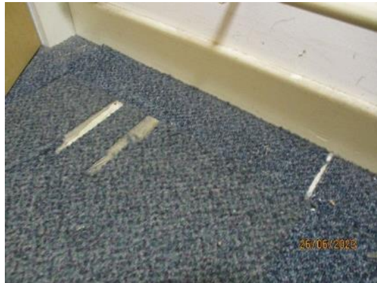
63. Carpet tiles damaged
