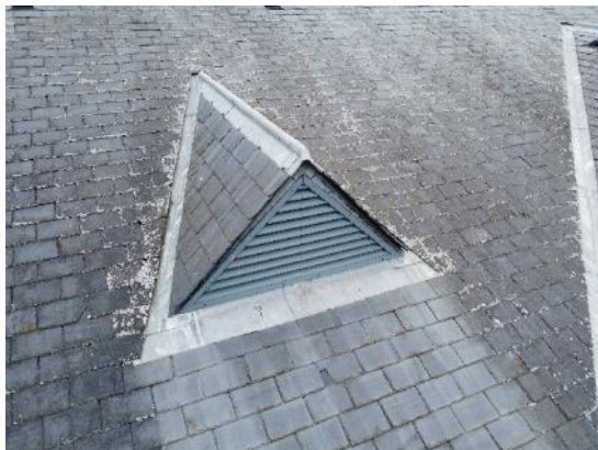
10. Isolated broken slates
