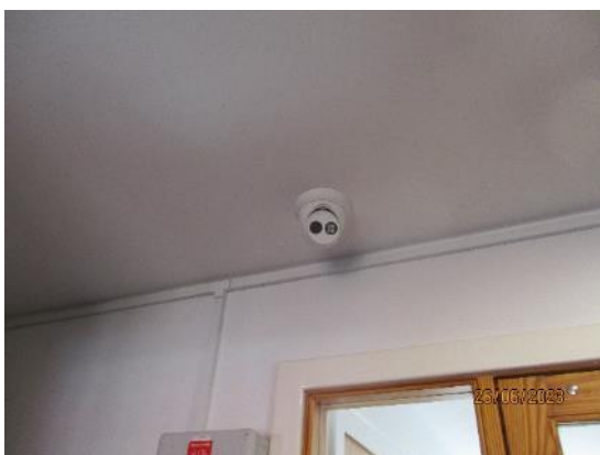
187. CCTV camera internal.
