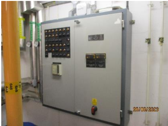
137. Heating and ventilation control panel. Plant room
