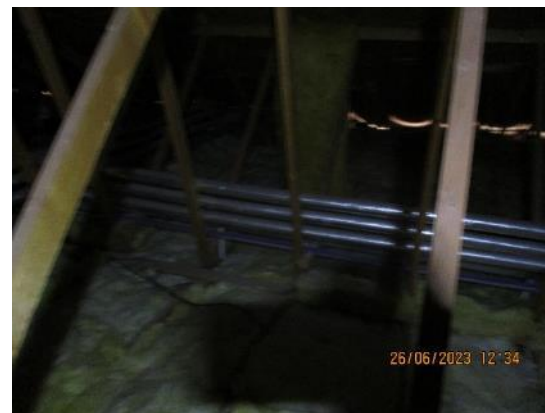
146. Pipework – cold water attic space.
