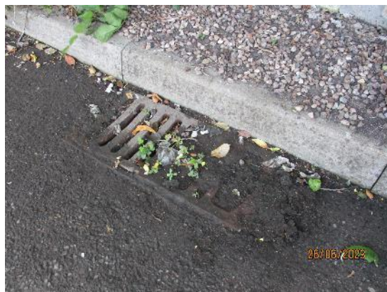
224. Car park road gully blocked
