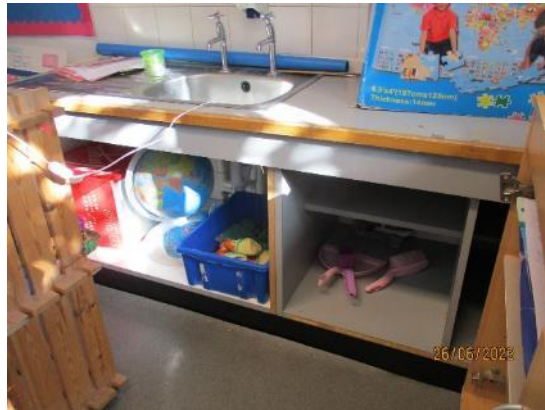
130. Base units missing doors
