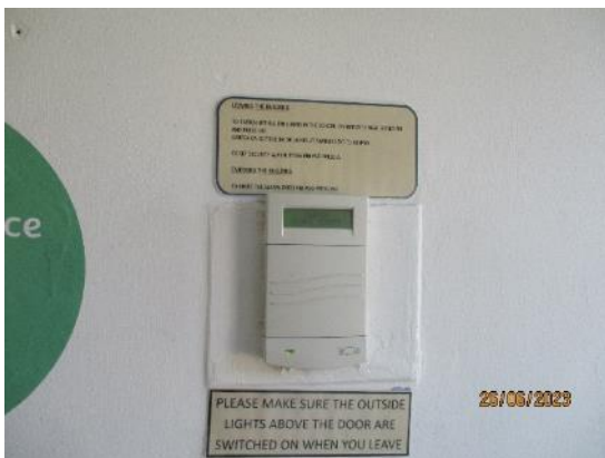
181. Intruder alarm system user control unit.
