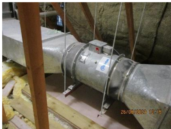
152. Toilet extract fan system attic space.
