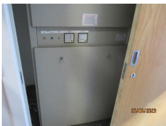
175. Emergency lighting central battery
