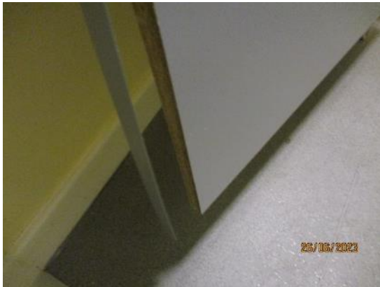
112. Edging coming loose
