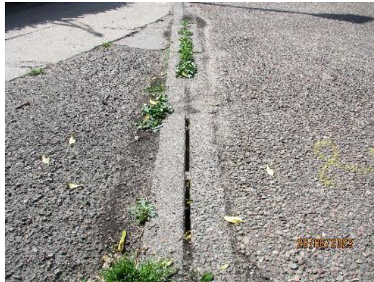
222. Concrete channel drain blocked
