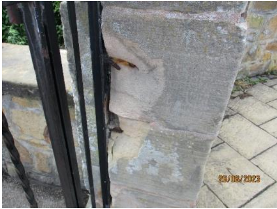
213. Masonry damage and erosion
