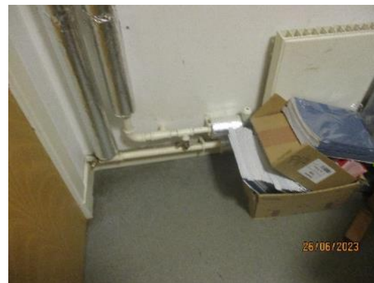
140. Pipework heating system typical internal.
