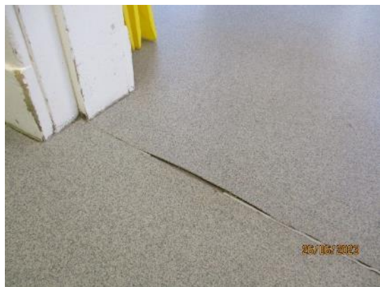
59. Edges lifting, seam joints failed
