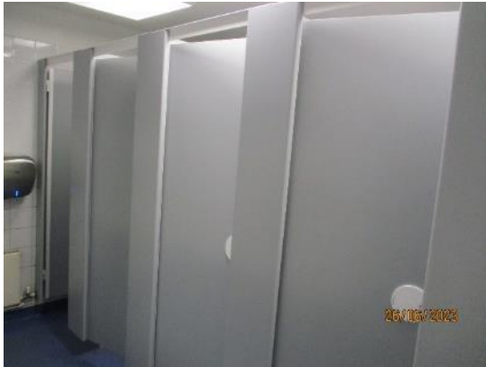
110. Composite panel cubicle partitions
