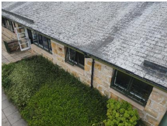
21. Missing section of snow boards
