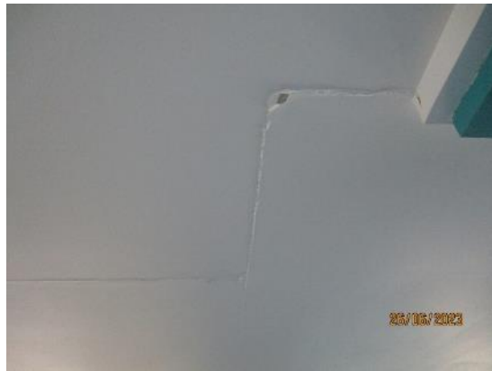
72. Cracking at joints
