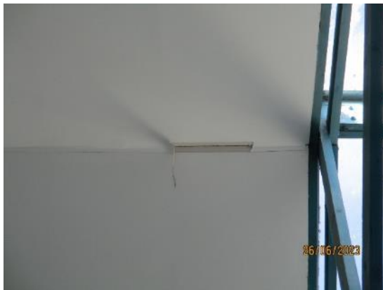
73. Failed taped joints
