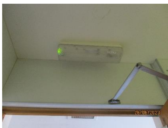
176. Emergency lighting boys toilets.
