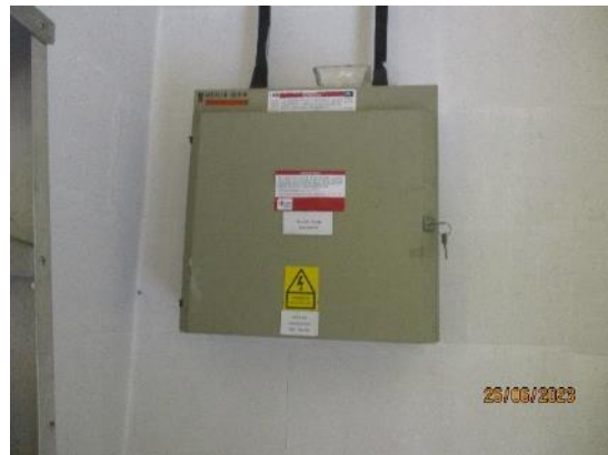
162. DB – LP plant room.
