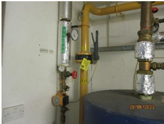
147. Gas pipework plant room typical.
