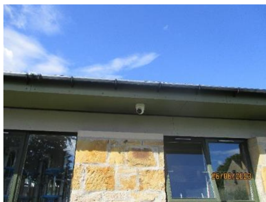
188. CCTV camera East end entrance.
