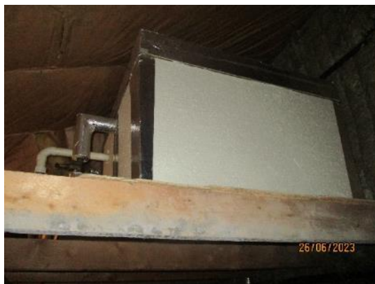
139. Heating feed and expansion tank attic space
