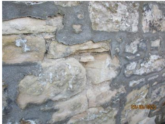
216. Spalling cement mortar pointing
