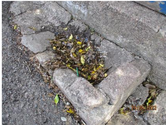
221. Drainage gully broken and blocked
