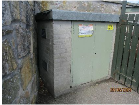
226. Gas meter house
