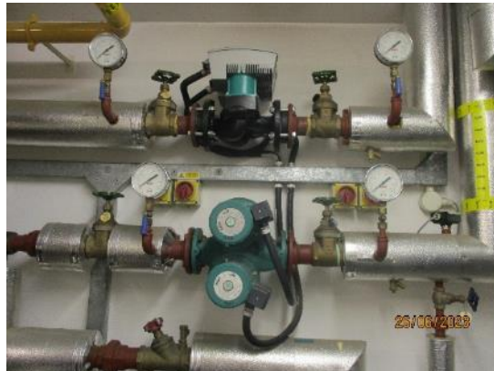
138. Pumps and pipework – heating system
