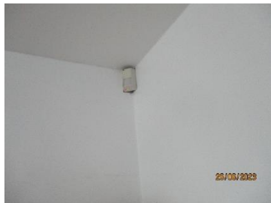
182. Intruder alarm system PIR.
