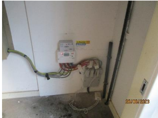
166. Incoming power supply and hydro fuses 1/11a
