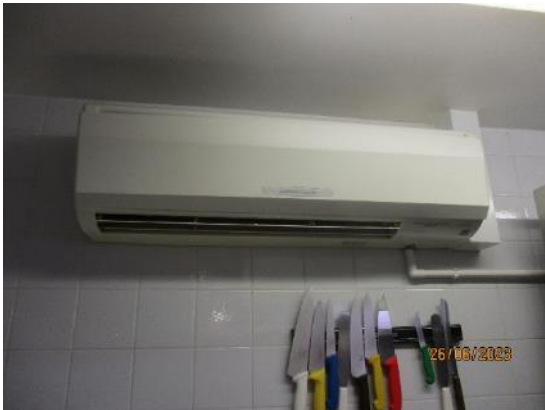
155. Air conditioning indoor unit kitchen.
