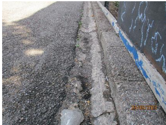
220. Concrete channel drain cracked and broken
