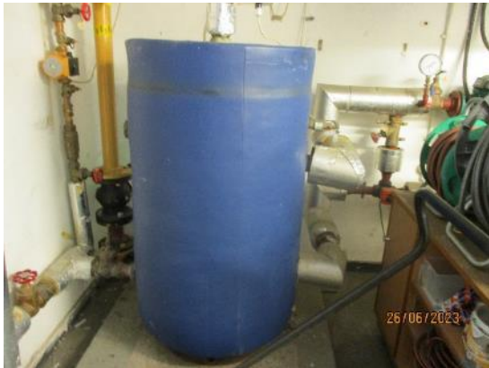
143. Hot water calorifier plant room.
