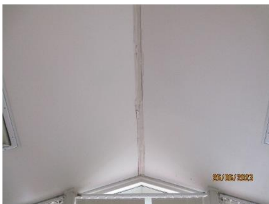
75. Failed taped joints
