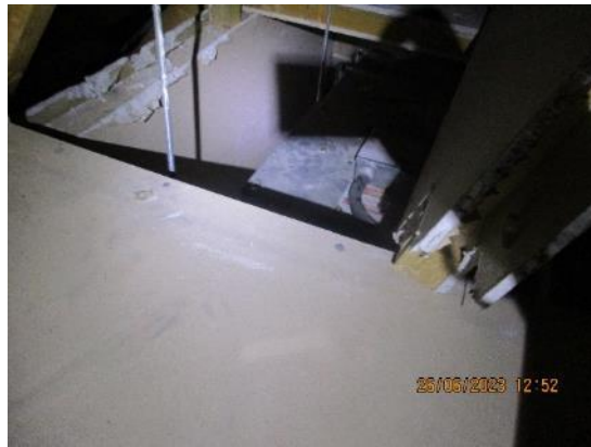
154. Kitchen air handling unit attic space.
