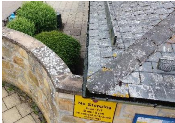
28. UPVC gutters with standing water
