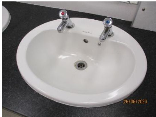
106. China vanity basins – Boys toilets
