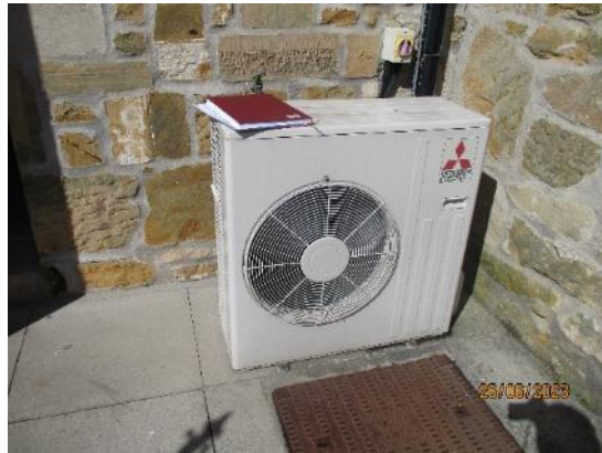
156. Air conditioning outdoor unit kitchen.
