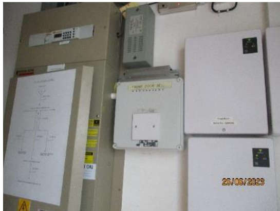
159. DB LP 1 – Electric cupboard 1/11a
