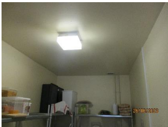
169. Lighting – stores typical.
