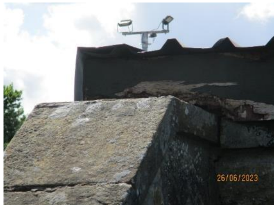
22. Rotten fascia board to external store
