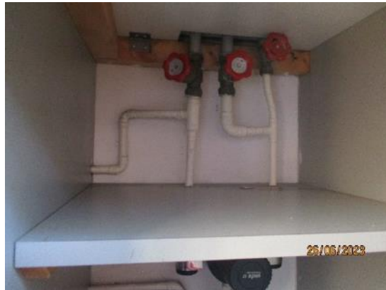
144. Pipework – hot water system typical.
