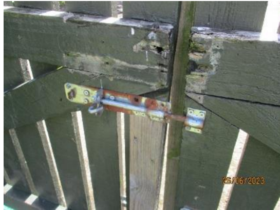
208. Damage and rot to timber gates
