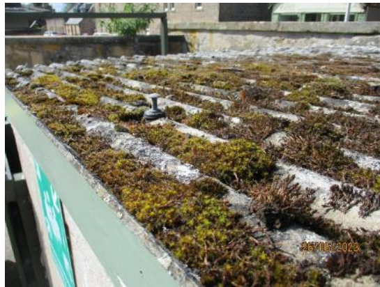
14. Corrugated asbestos roof (salt store)
