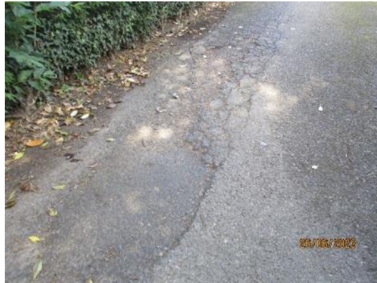
190. Cracked and pot holed
