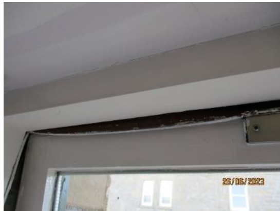
44. Seals to frames failing
