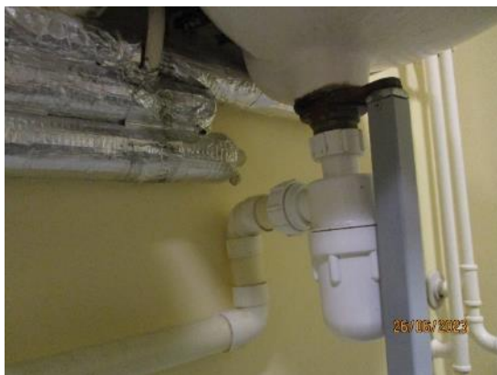
108. PVC waste pipes
