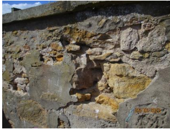
214. Eroded, crumbling masonry
