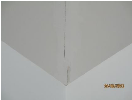
71. Cracking at taped joints
