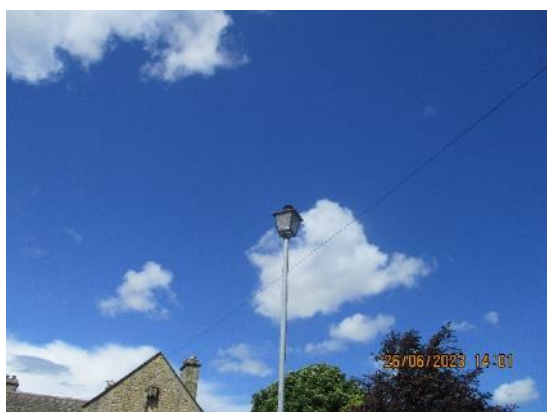
173. External car park lighting.
