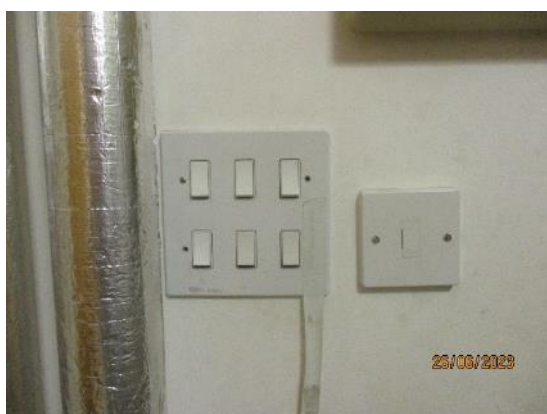
171. Light switch control typical.
