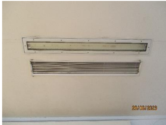
168. Lighting – sports hall.
