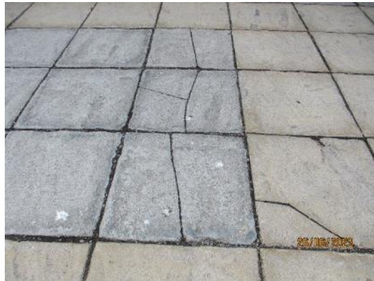
198. Cracked, loose and uneven slabs
