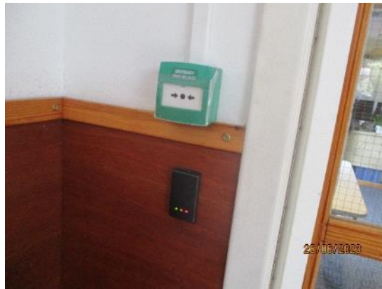
184. Security door card reader and emergency release unit typical.
