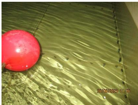
145. Cold water storage tank internal view attic space
