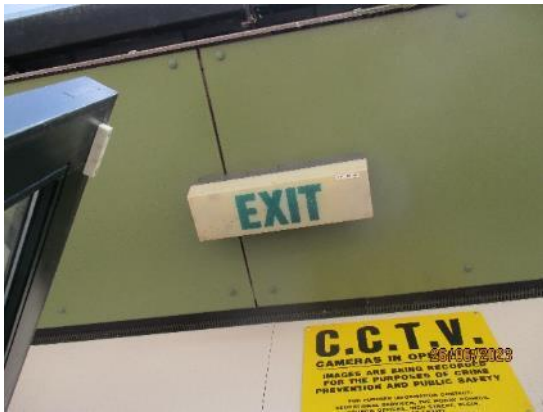
177. Emergency exit sign light front door.
