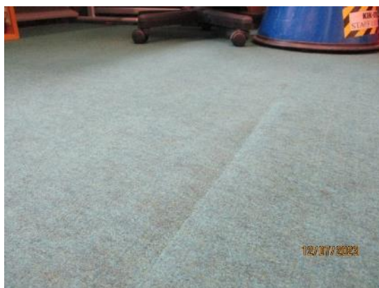
118. Uneven timber floor boards
