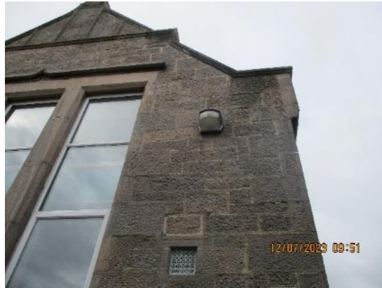
277. External building lighting typical.
