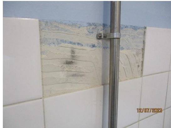
163. Missing ceramic tiles
