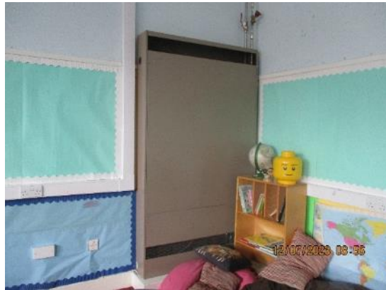
231. Heating system fan convector heater.
