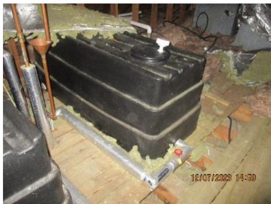
244. Cold water storage 2 tank kitchen attic.
