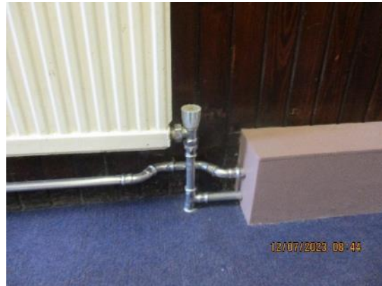
237. Pipework – heating system.
