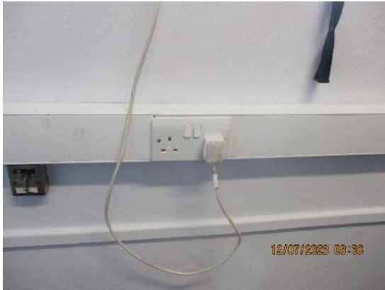
264. Socket and dado trunking typical.
