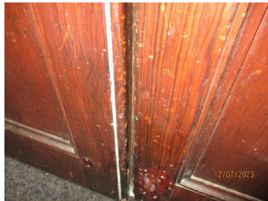
175. Gaps between door leaves
