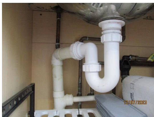
211. PVC waste pipes
