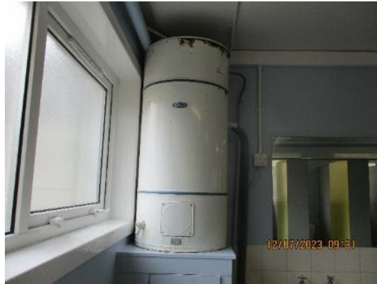
241. Hot water storage tank girls toilets.
