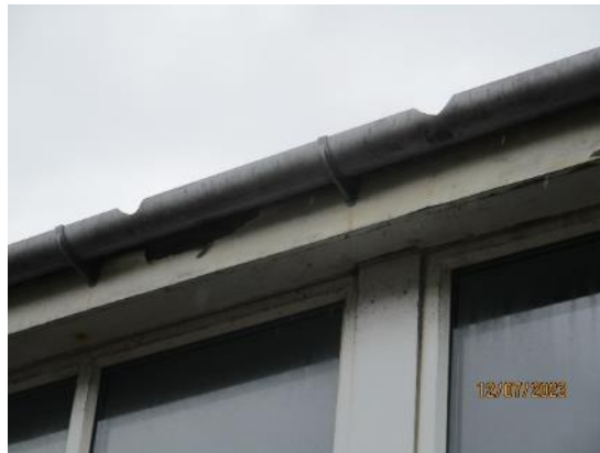
44. Broken upvc gutter
