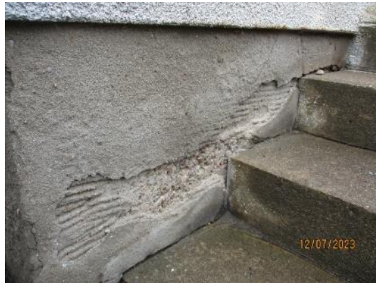
87. Spalling smooth render to Dining Hall
