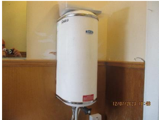
243. Point of use water heater upstairs toilet.
