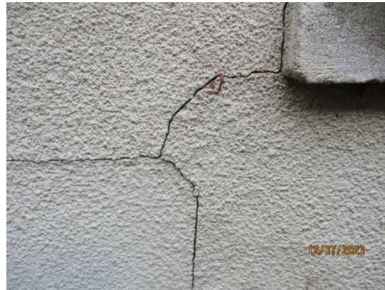
81. Cracked roughcast to school
