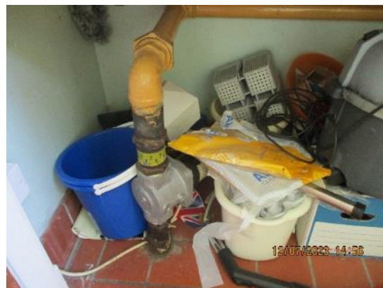
251. Gas solenoid valve. Kitchen supply.
