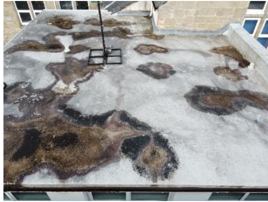
14. GRP blistered and uneven
