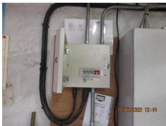
263. Electrical – DB basement plant room.
