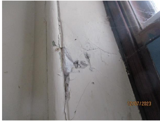
155. Damaged lath & plaster
