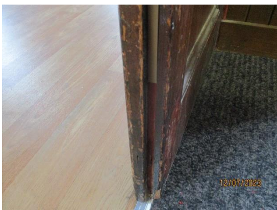
176. Missing intumescent strips
