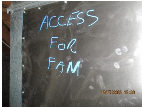
255. Kitchen canopy extract fan in ductwork in kitchen attic.
