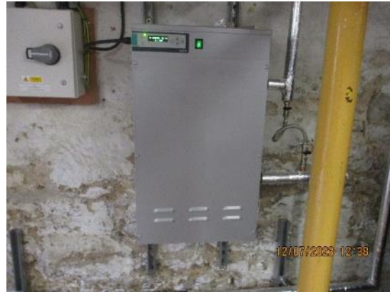
235. Heating system pressurisation unit 0/1
