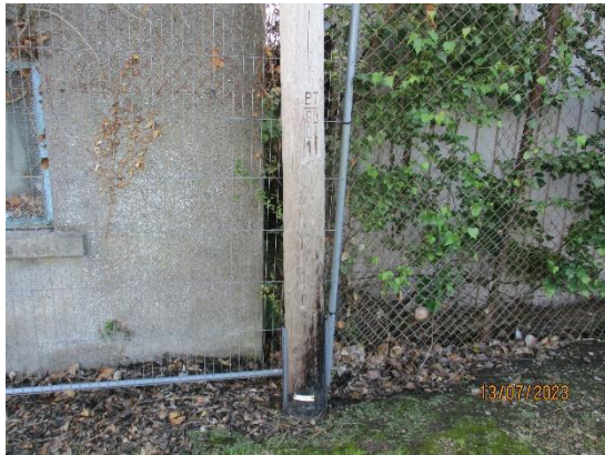
350. Timber utility pole (BT)
