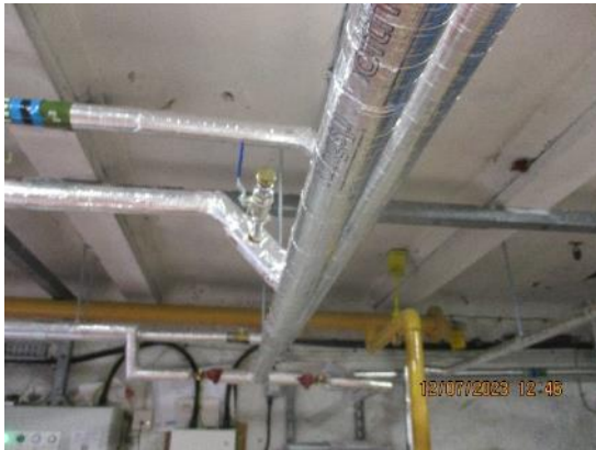
236. Pipework – heating system 0/1
