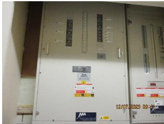
259. Electrical main DB – 1/10.
