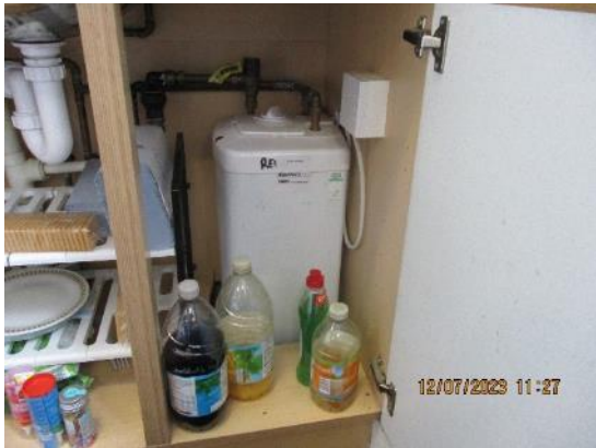
242. Point of use water heater. Main school.
