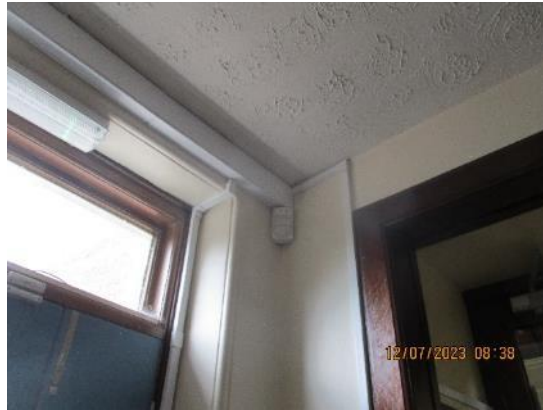
289. Intruder alarm system motion sense detector.
