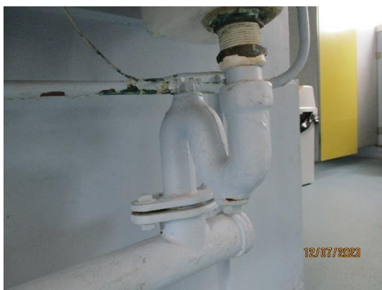
201. Cast iron waste pipes (Girls toilet)
