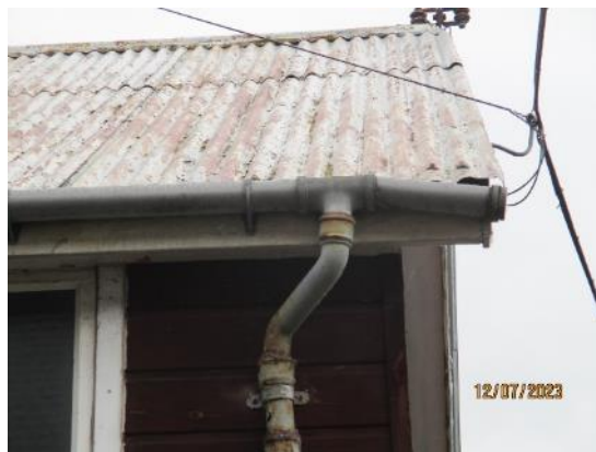
42. Unsupported upvc gutter
