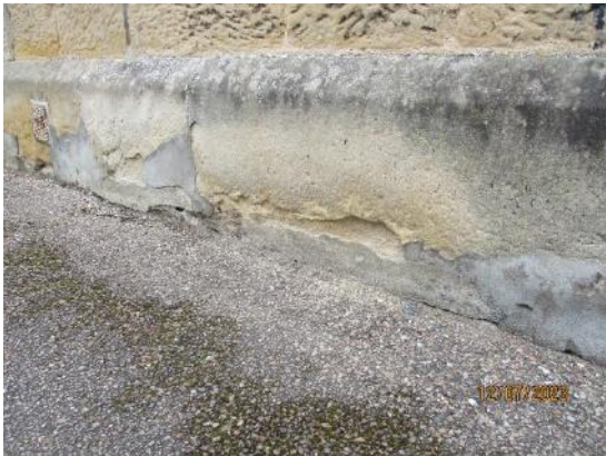
80. Surface erosion of stone walls
