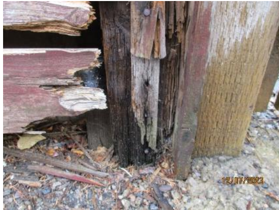
67. Rot in timber frame to Hut
