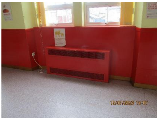
232. Heating system fan convector dining room.
