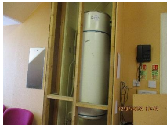
239. Hot water storage tank staff room.
