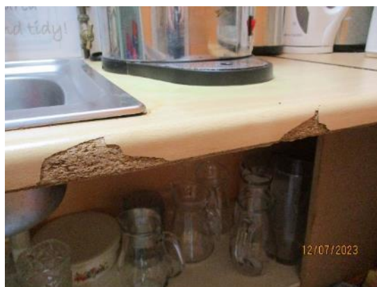
225. Chipped and water damaged worktops
