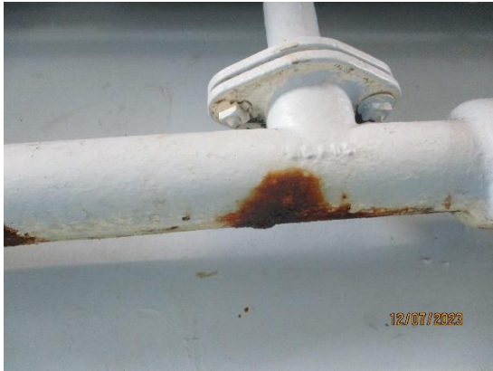
202. Leaking cast iron waste pipes
