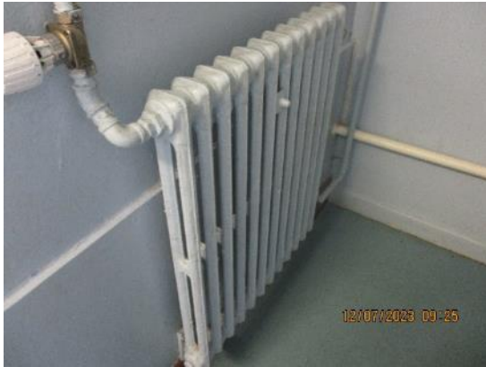
234. Radiator cast iron – boys toilets.
