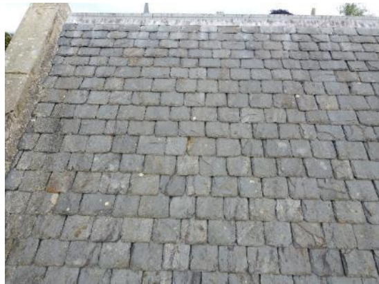
20. Chipped and broken slates
