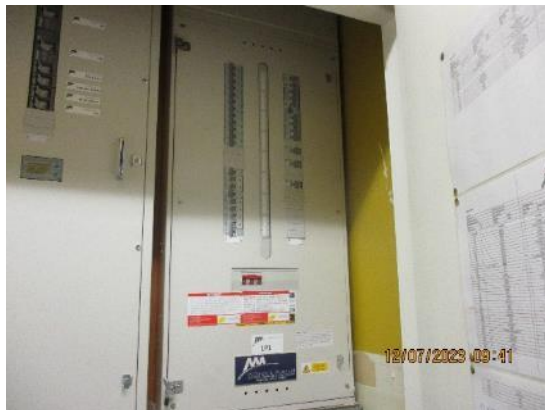
260. Electrical DB LP1 – 1/10
