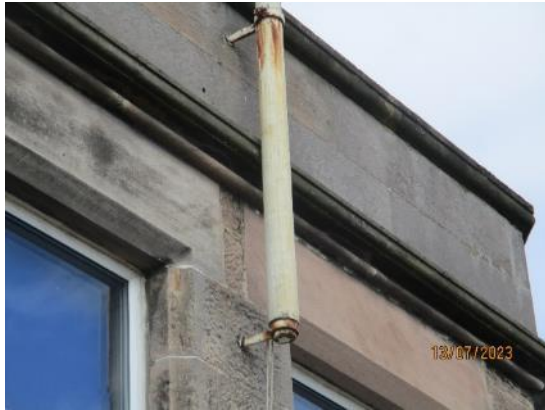
61. Corroded flag pole brackets
