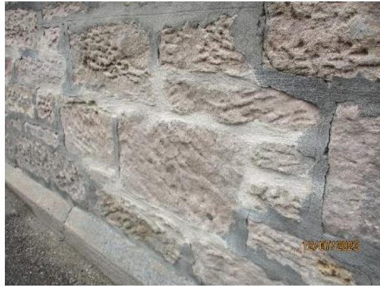
85. Poor pointing and erosion to Dining Hall
