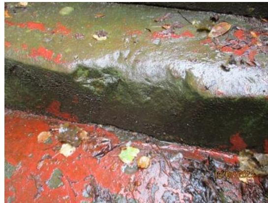
115. Damage to stone steps
