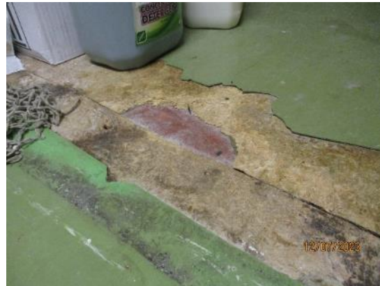
123. Cracked and lifting
