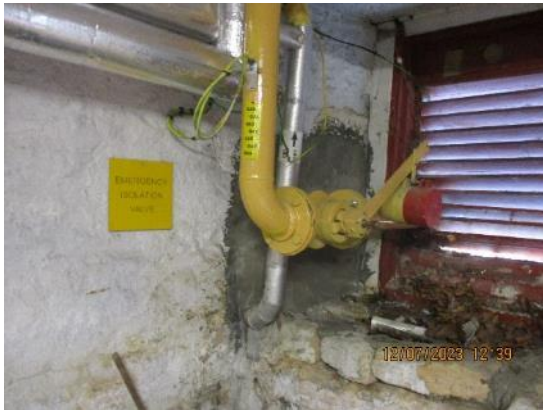
248. Gas pipework and shut off valve main school O/I.
