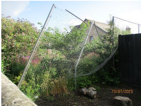
314. Damaged chain link fencing
