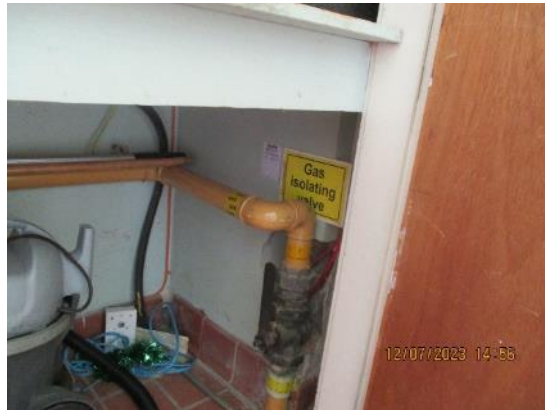
249. Gas pipework – kitchen incoming supply.
