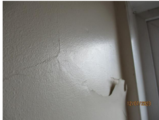
217. Peeling paint to lath & plaster walls
