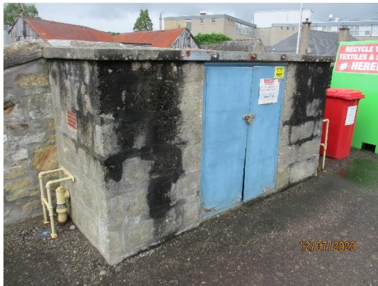
348. Gas meter house
