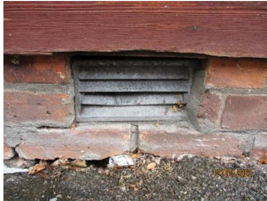
73. Underfloor ventilation to Hut
