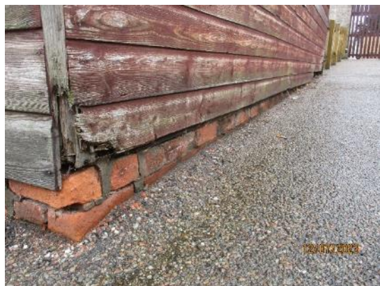
83. Rot and damage to timber linings
