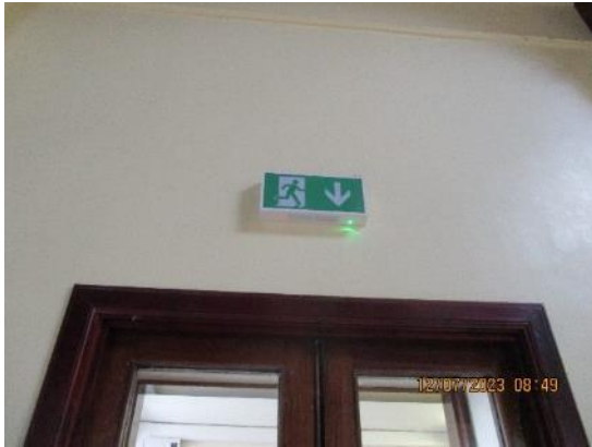
276. Emergency exit sign light typical.
