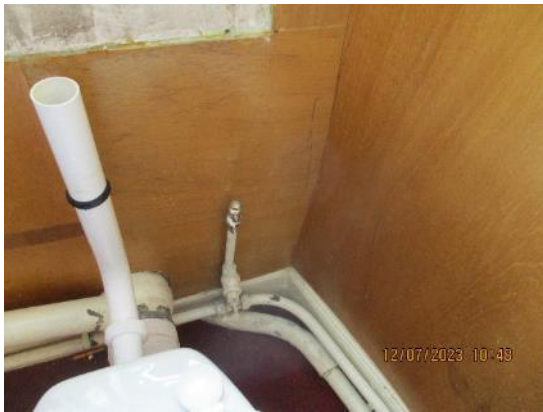
246. Pipework – cold water upstairs toilet.
