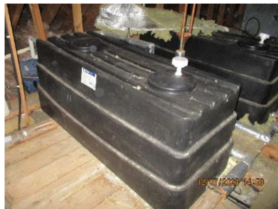
245. Cold water storage tank 1 kitchen attic.
