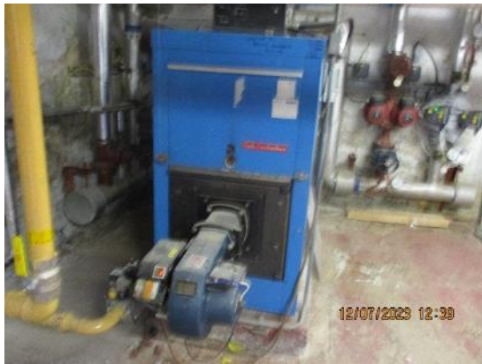
228. Gas boiler – basement plant room. 0/1
