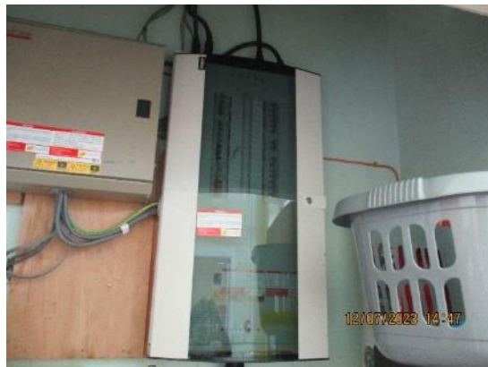
261. Electrical DBs – kitchen block cupboard.
