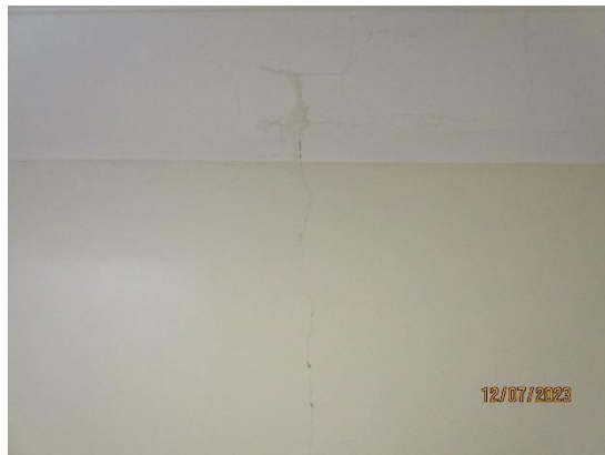
157. Cracked lath & plaster
