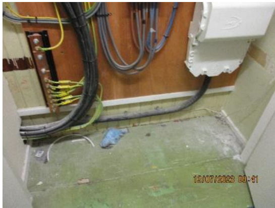
258. Electrical incoming supply and hydro fuses.
