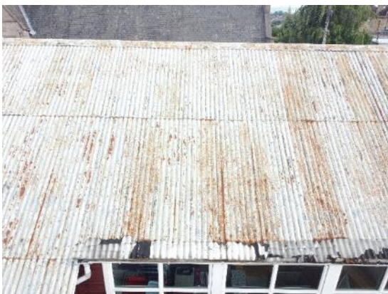
17. Corroded and damaged corrugated iron
