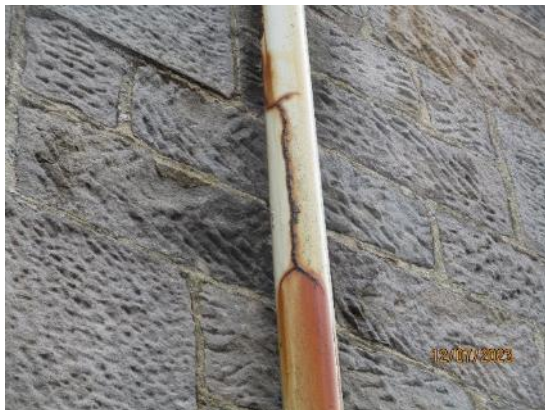
52. Cracked, leaking downpipes
