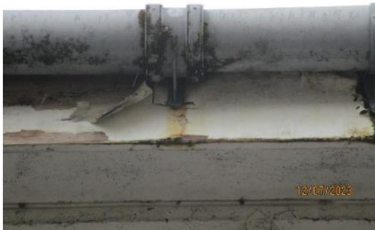
43. Leaking upvc gutters
