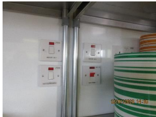
267. Isolation switches – kitchen.
