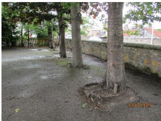
299. Tarmacadam damaged by tree roots
