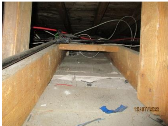
34. No insulation above Boys toilet
