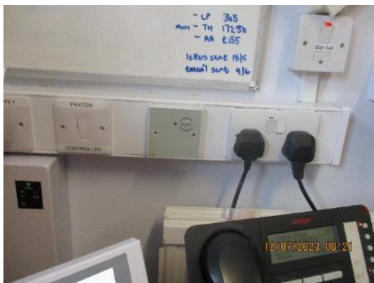
287. Disabled toilet alarm system alert panel in reception office 1/3 from 1/27.
