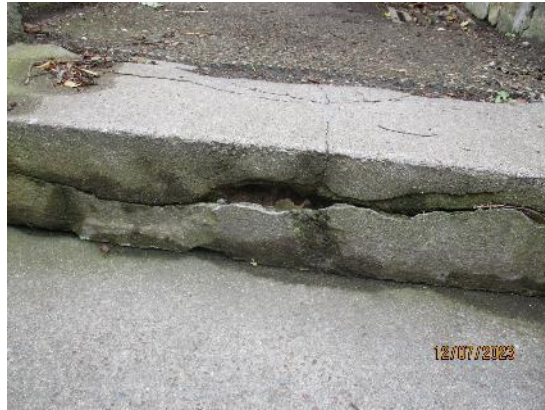
307. Damaged concrete steps
