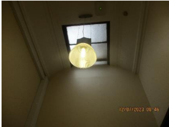
270. Lighting – corridor typical.
