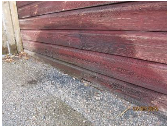
75. Ground level too high
