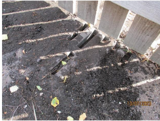
343. Silt blocking gullies
