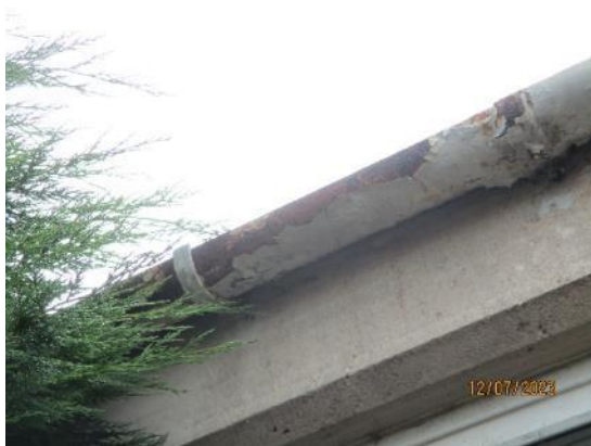
106. Peeling paint to cast iron rainwater goods
