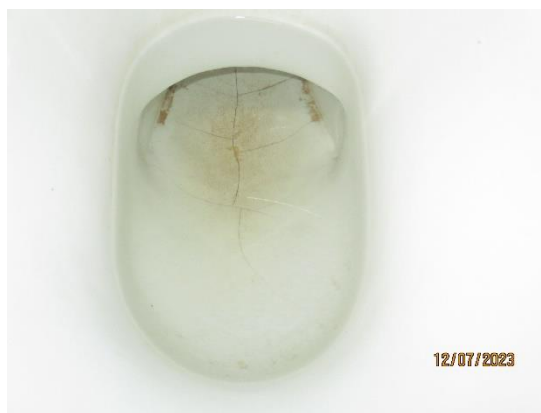
195. Cracked sanitary ware
