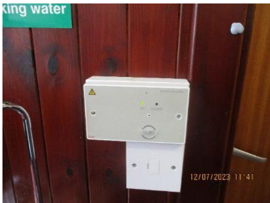
286. Disabled toilet alarm system DPT 1/27.
