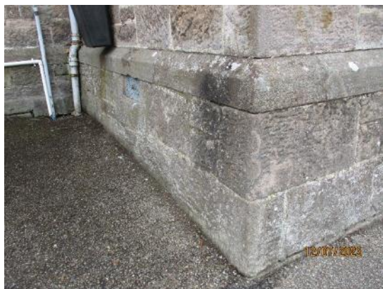
71. Underfloor ventilation to school building
