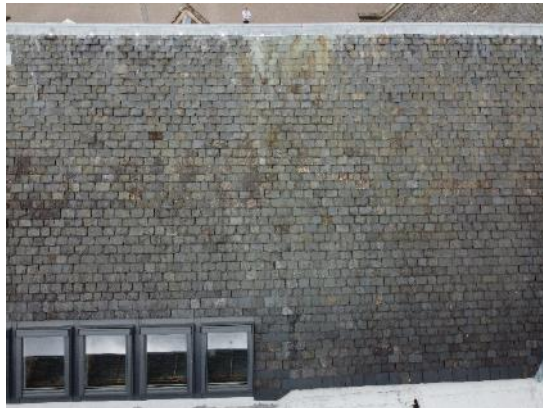
9. Slates are dated but in fair condition
