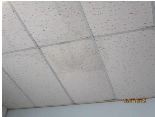
144. Damaged, sagging ceiling tiles
