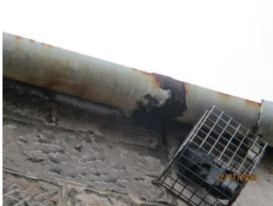
37. Leaking cast iron gutters
