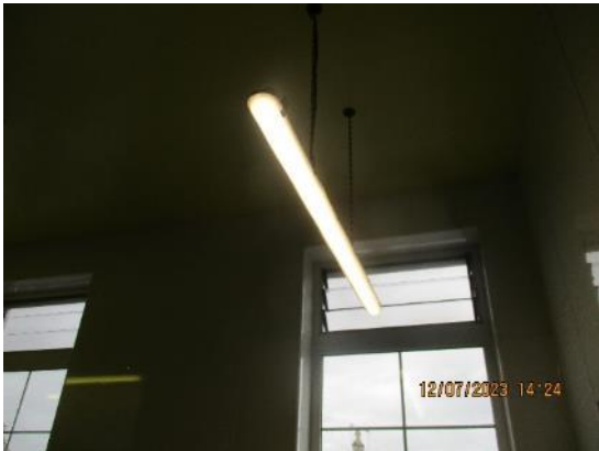
272. Lighting – main kitchen.
