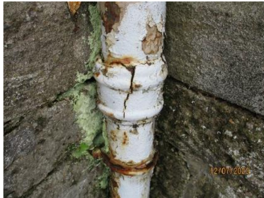
46. Cracked, leaking cast iron downpipes
