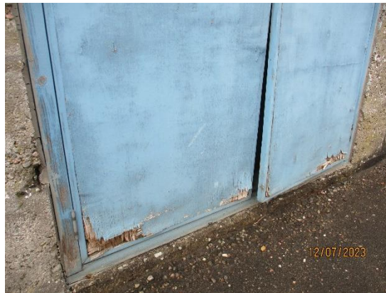
349. Rotten, twisted timber doors
