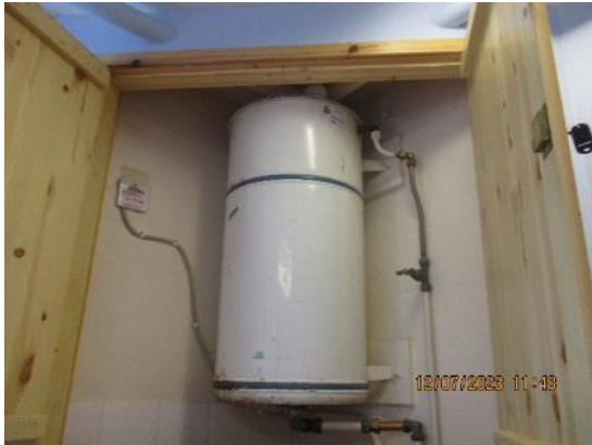
240. Hot water storage tank boys toilets 1/28.
