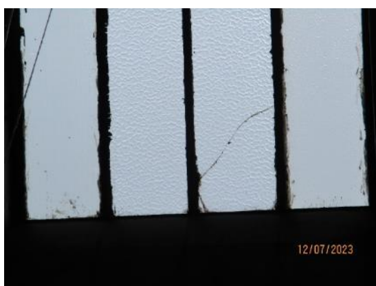
29. Metal skylights with broken glass
