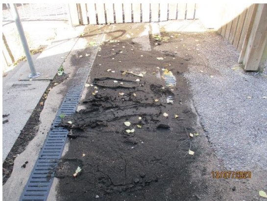
341. Silt blocking drainage
