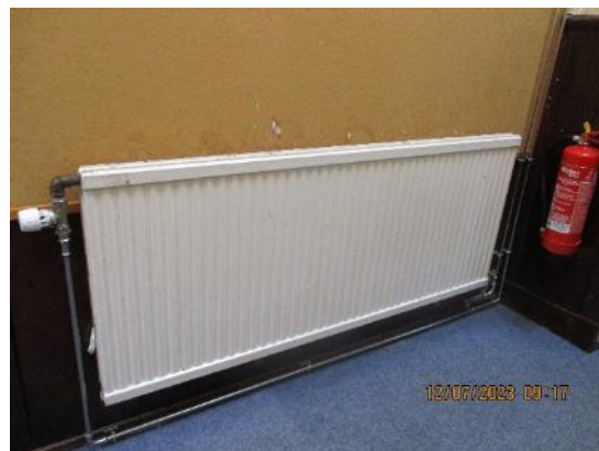
233. Radiator – steel panel typical.
