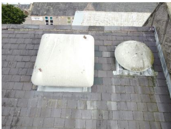
256. Kitchen canopy fan terminal on roof.
