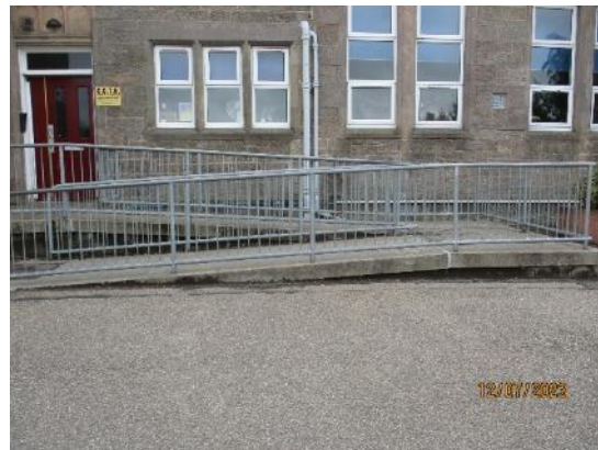
117. Galvanised guardrails to ramps
