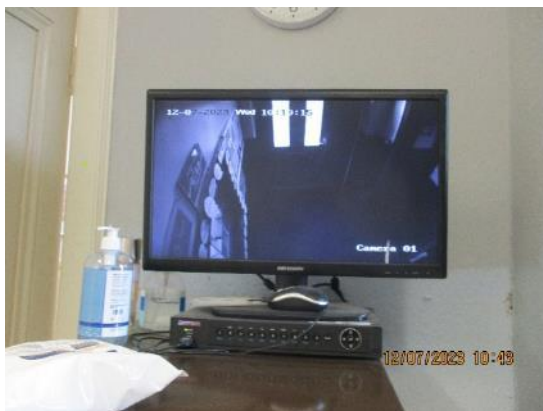
293. CCTV monitor and recorder HT office.
