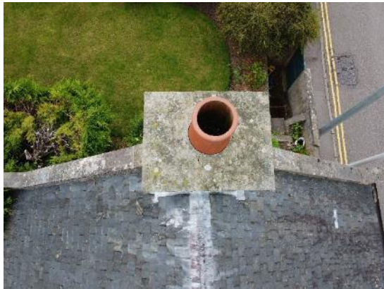
57. Clay pot not capped and vented
