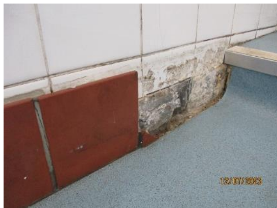
131. Broken/missing quarry tile skirting
