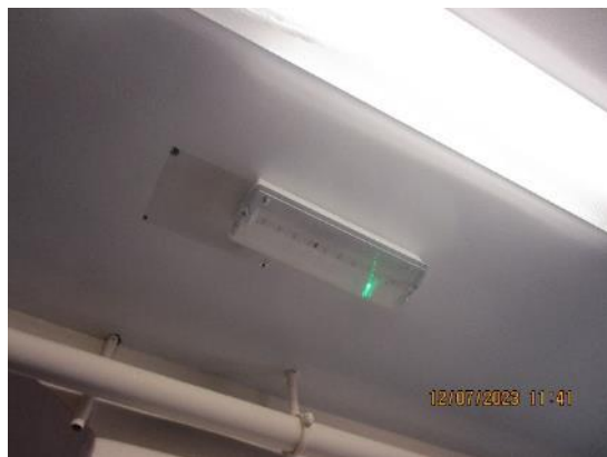
275. Emergency lighting dedicated bulkhead. LED
