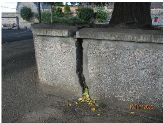
311. Damaged tree planters
