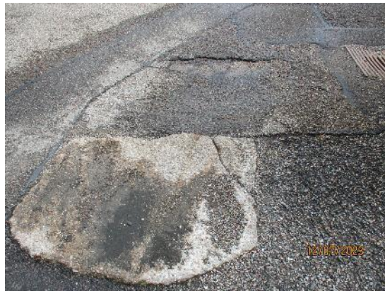
295. Potholes and patches
