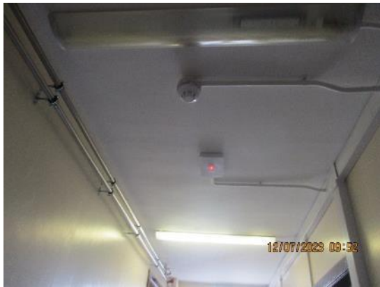
282. Smoke detector/sounder typical.
