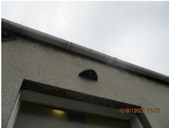
278. External building lighting kitchen block.
