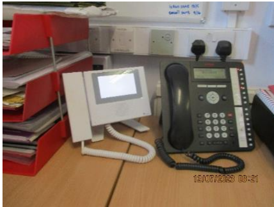
291. Paxton main entrance door security monitor and control handset reception office 1/3.
