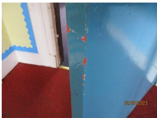
220. Chipped paint to timber doors
