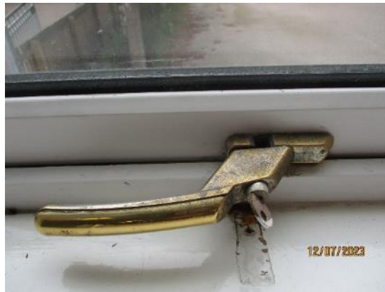
103. Surface damage to ironmongery
