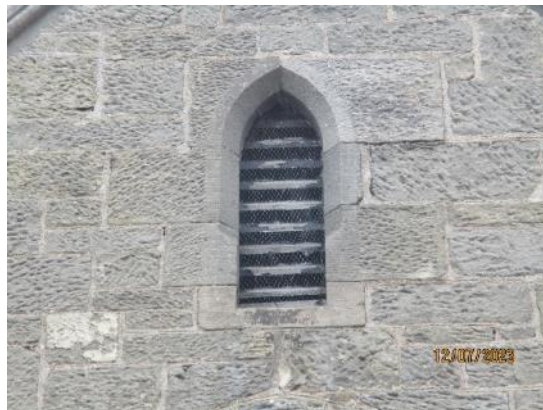
105. Peeling paint to louvered window vents
