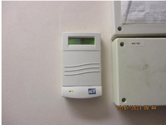
288. Intruder alarm user control keypad.
