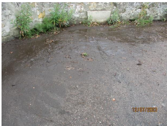
340. Silt from surface flooding
