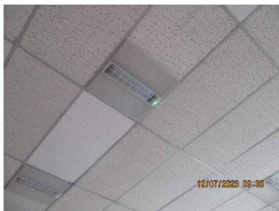
269. Lighting – classroom typical.
