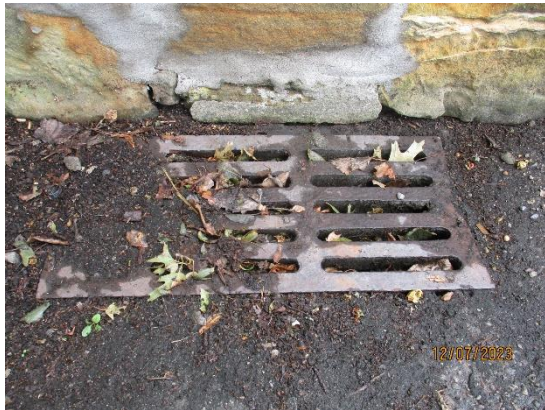
339. Blocked playground drainage
