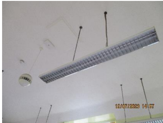
273. Lighting – dining room.
