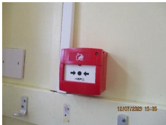
281. Fire alarm call point.
