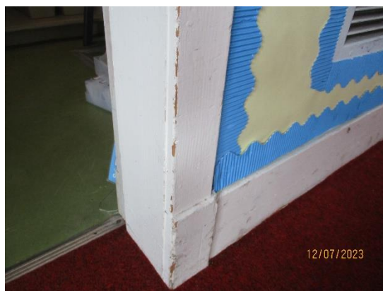
221. Chipped paint to joinery items
