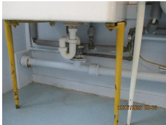
247. Pipework – hot and cold girls toilet.
