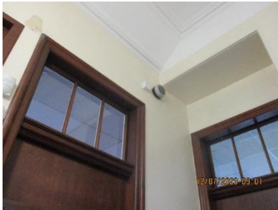
285. Period bell – corridor typical.
