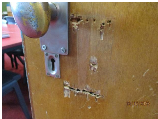
171. Damaged timber hollow core doors
