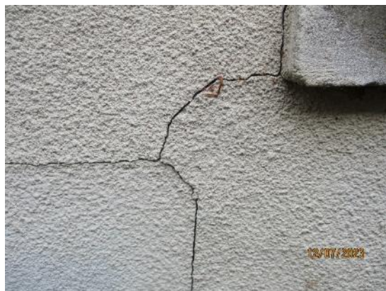
65. Cracked masonry walls
