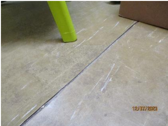
122. School – Linoleum in cupboards etc
