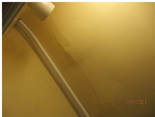
142. Cracked lath & plaster ceilings
