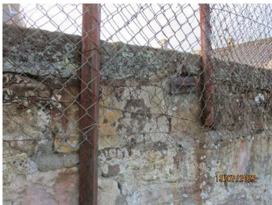
316. Corroded chain link posts
