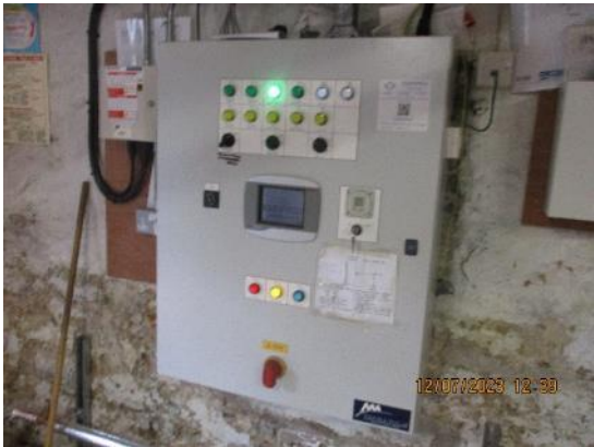
230. Heating control panel 0/1
