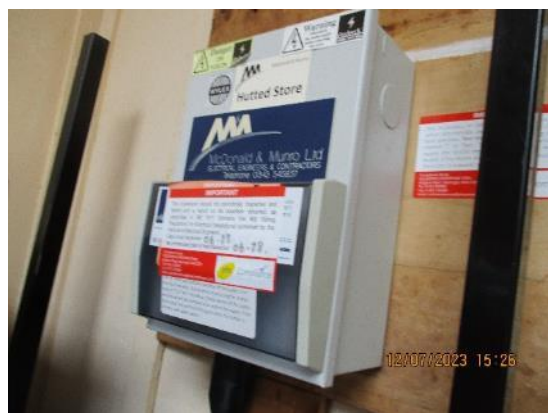
262. Electrical consumer unit hutted store.
