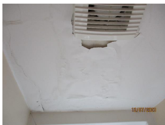
212. Peeling paint to ceilings
