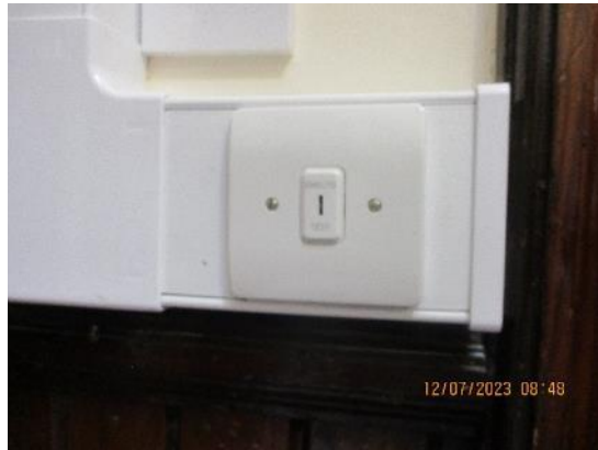
279. Emergency light test switch typical.
