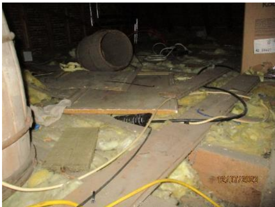
33. Displaced mineral fibre insulation
