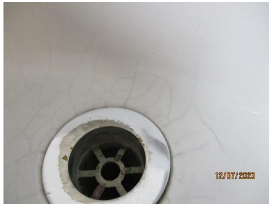
197. Cracked china basins
