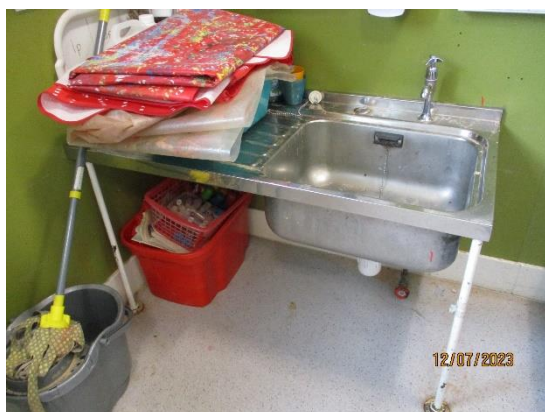
208. Stainless steel classroom sinks
