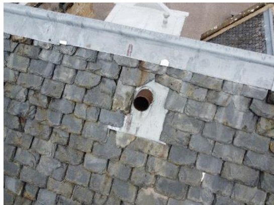
10. Isolated missing/damaged slates
