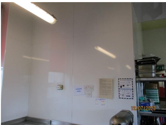
164. Wetwall in Kitchen
