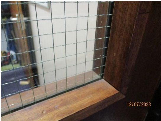
186. Georgian wired glass to fire doors
