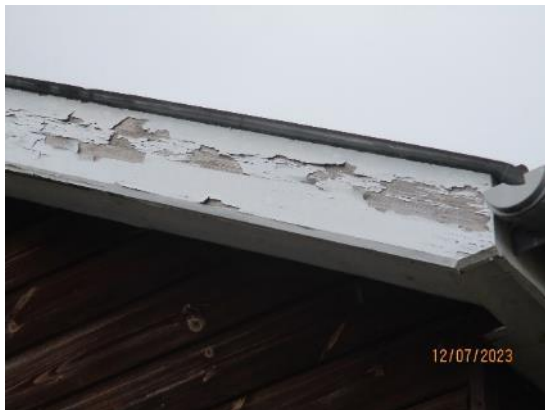
104. Peeling paint to barge boards
