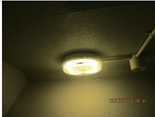
271. Lighting – stores typical.
