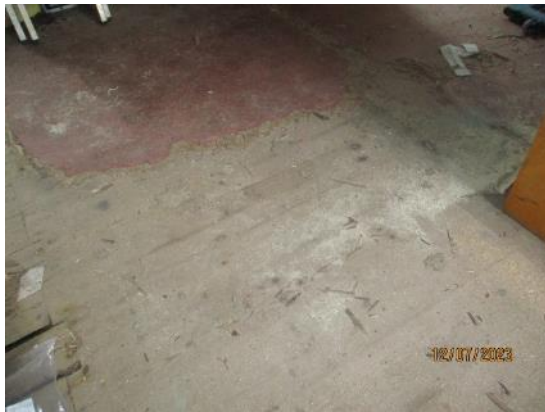
132. Damaged linoleum in the Hut
