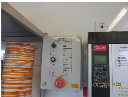
250. Gas safety control panel – kitchen interlock.
