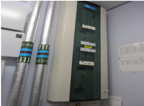
233. Distribution board nursery utility room GO5
