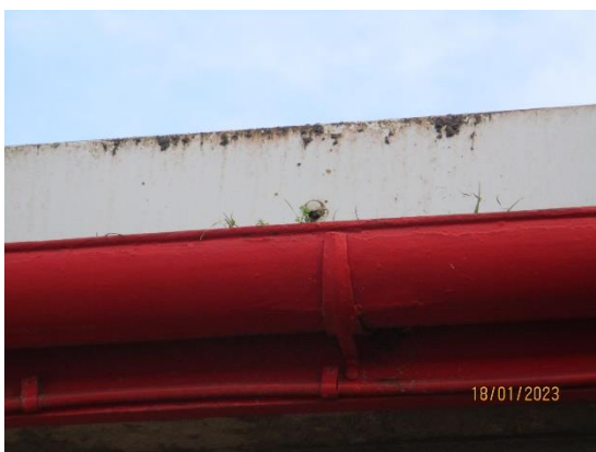
29. Vegetation in gutters
