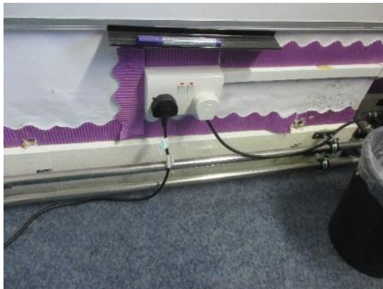
237. Sockets main school typical
