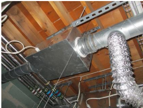
225. Heat recovery ventilation unit. Nursery toilets G05
