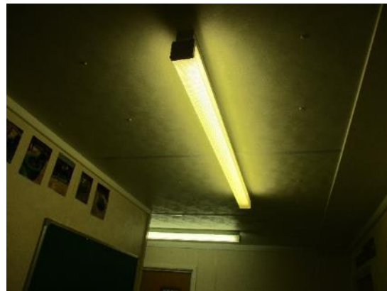
252. Lighting – ASN corridors typical
