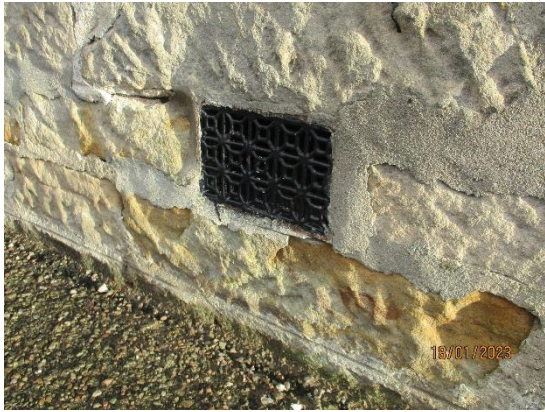
43. Ventilation to stone building
