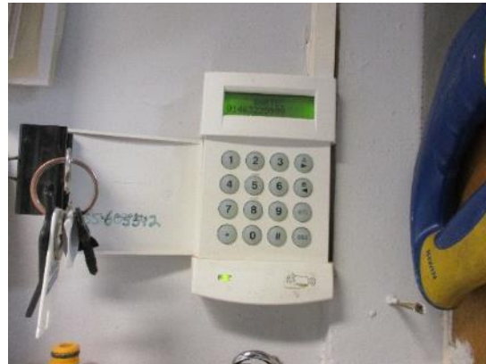
276. Intruder alarm keypad main school room 1/2
