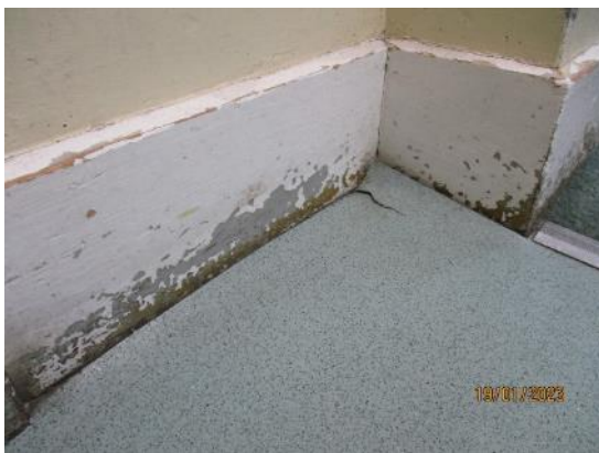
191. Paint chipped and peeling on joinery items
