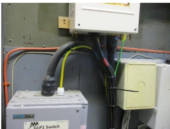
241. LV cabling – 1/3 meter cupboard main school
