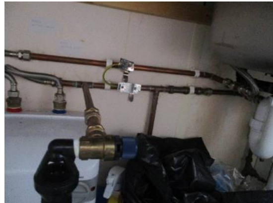
216. Pipework – hot and cold in ASN building typical.
