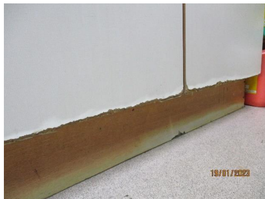
197. Damaged sink base units
