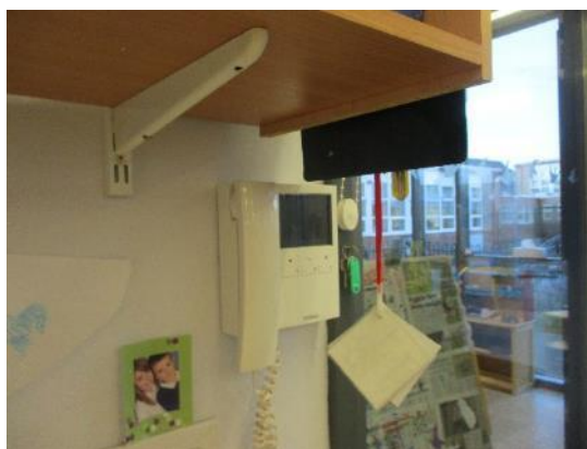
280. Door access control handset – nursery.
