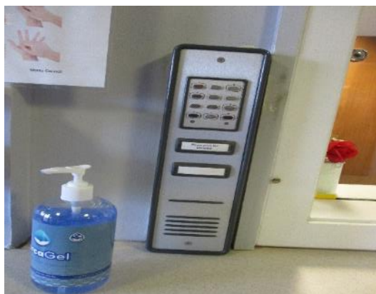
281. Door access intercom – Main school reception for internal entrance door.
