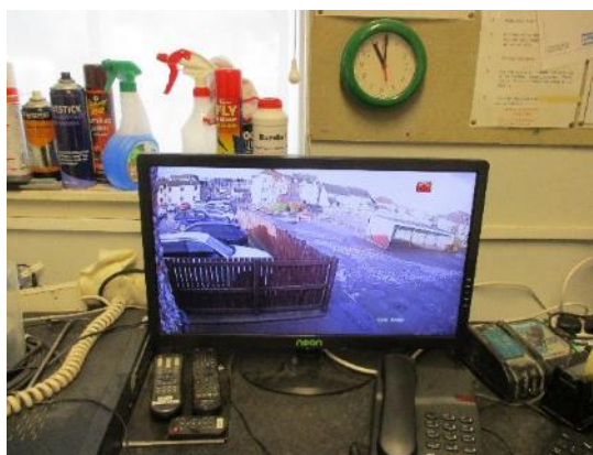
284. CCTV monitor and recorder main school 1/2
