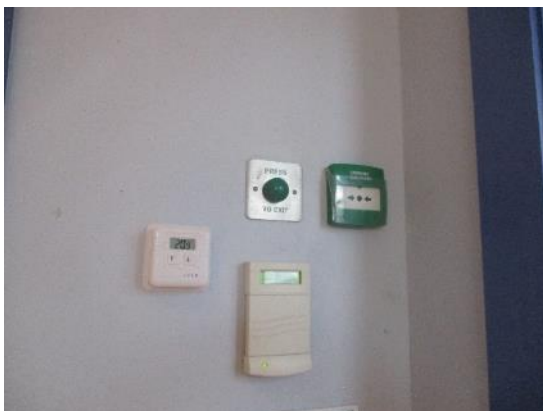
277. Intruder alarm keypad – Nursery extension.
