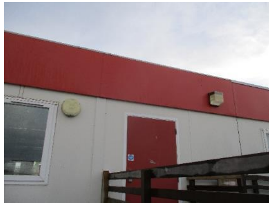
262. External lighting – ASN building example
