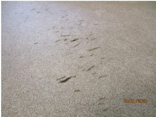
88. Surface damage to vinyl flooring
