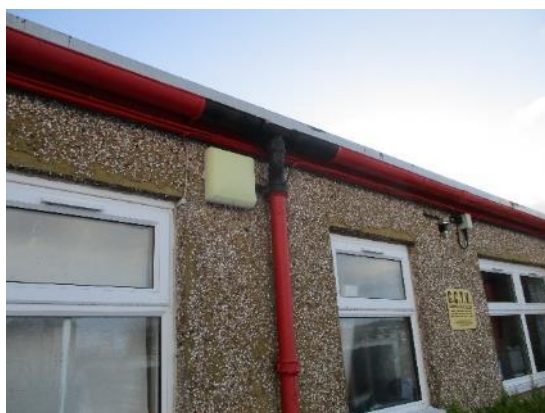
260. External emergency light main school entrance
