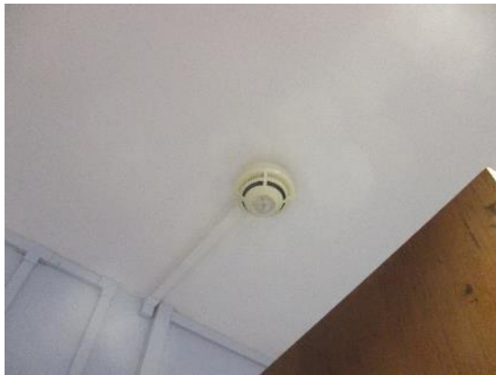
267. Fire system detection head – main school and ASN building typical
