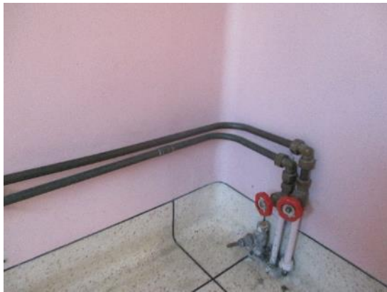
213. Pipework – hot and cold existing. Main school 1/63
