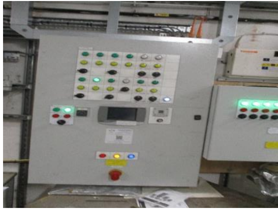
202. Control panel – heating. 0/71
