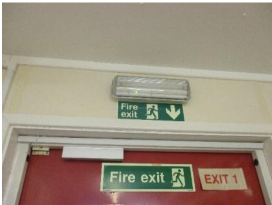
257. Emergency lighting ASN building typical exit.
