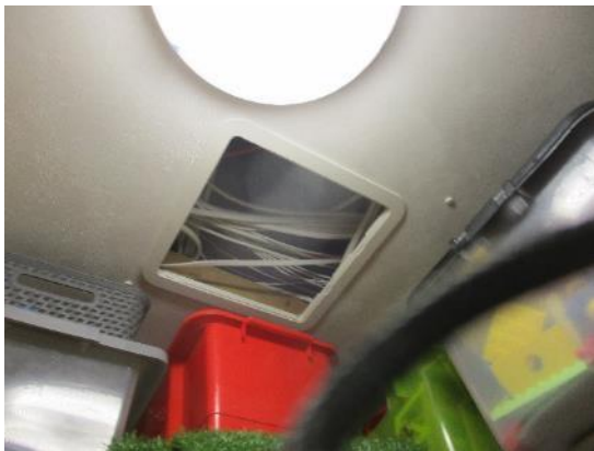
239. General wiring – ASN building ceiling space.
