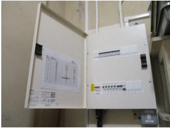
231. Distribution board main school 1/60
