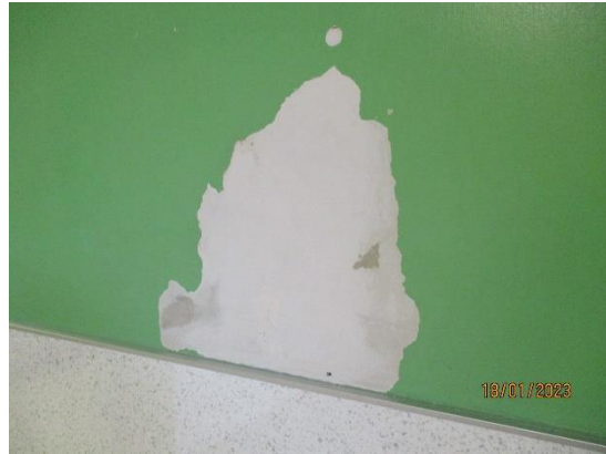
188. Paint peeling from plastered walls
