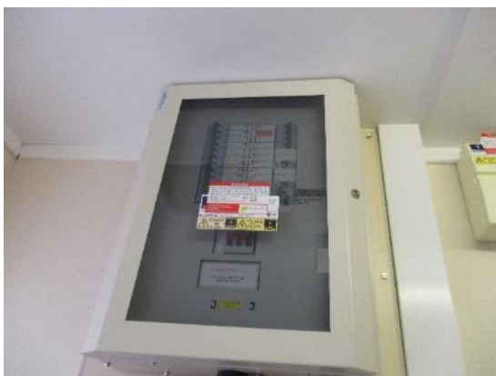
235. Distribution board – ASN building 1/79
