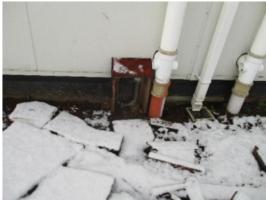
287. Cold water supply pipework ASN building.
