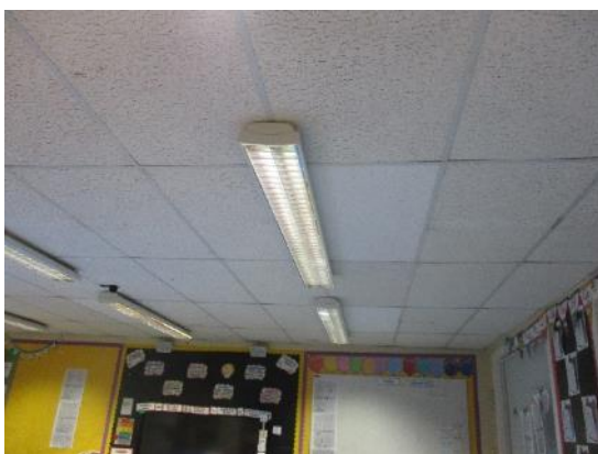
247. Lighting main school class typical
