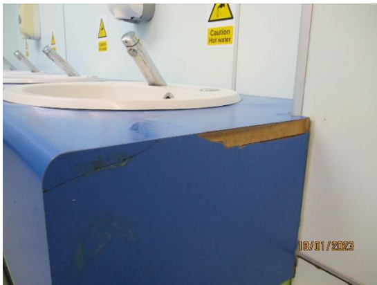
177. Damaged vanity units
