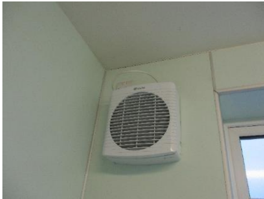
221. Extract fan 1/17 boys toilets main school
