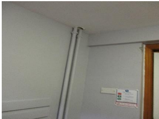
288. Pipework – heating system.
