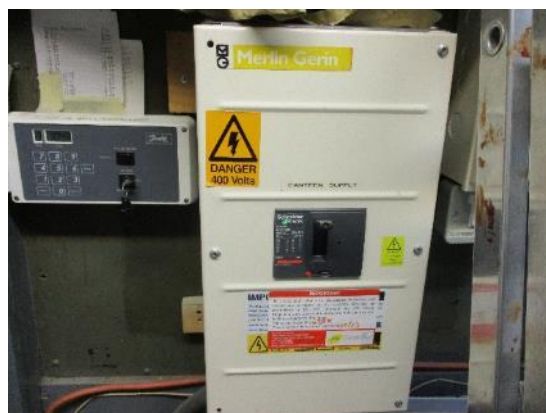
230. Main switch for canteen. Main school 1/3
