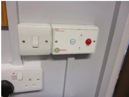
273. Disabled alarm system remote indicator. Main school reception office
