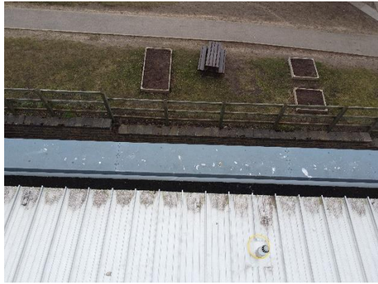
32. Part blocked gutter to New Nursery
