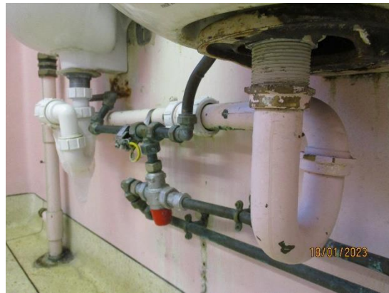
170. Copper and PVC waste pipes
