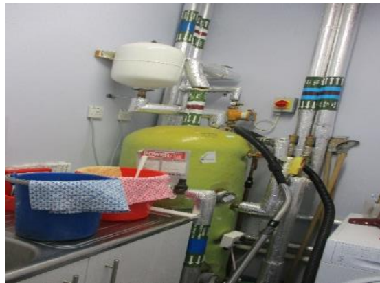
214. Hot water tank and pipework. Nursery GO2 utility.
