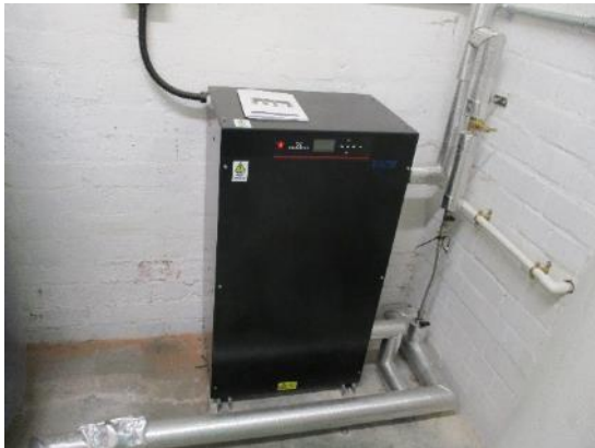
203. Pressurisation unit – heating – 0/71
