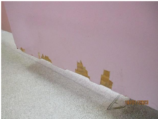
175. Damaged cubical partitions
