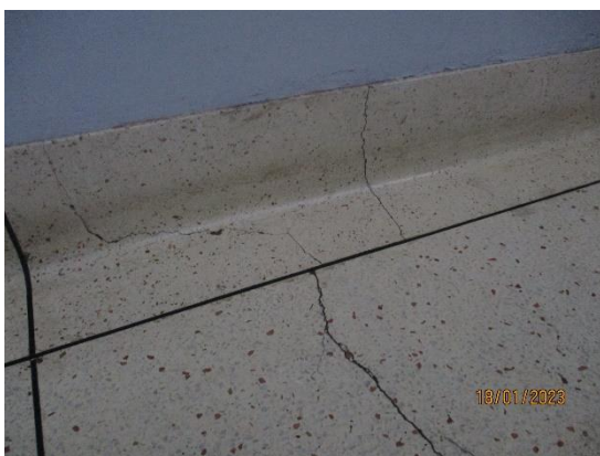
96. Cracked Terrazzo flooring
