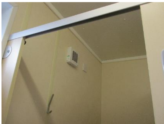
223. Extract fan ASN building typical 1-67 toilets
