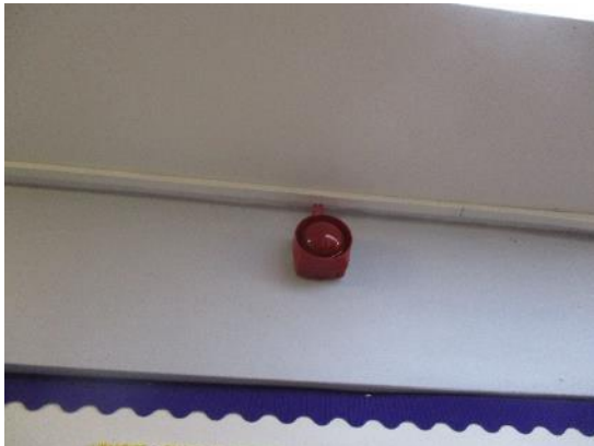
269. Fire detection system – strobe device typical.
