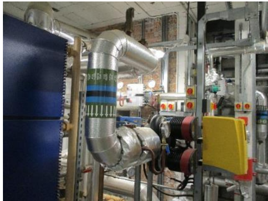
204. Pipework – heating system. 0/71
