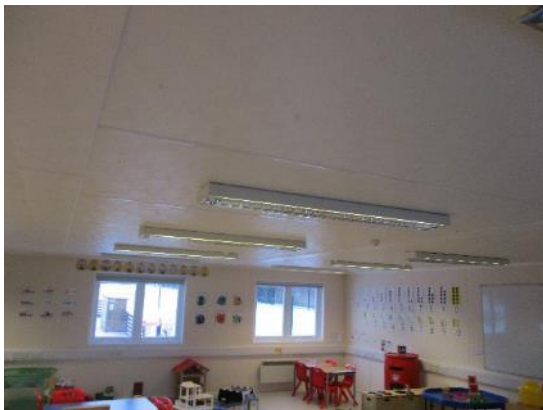
251. Lighting ASN building typical classroom
