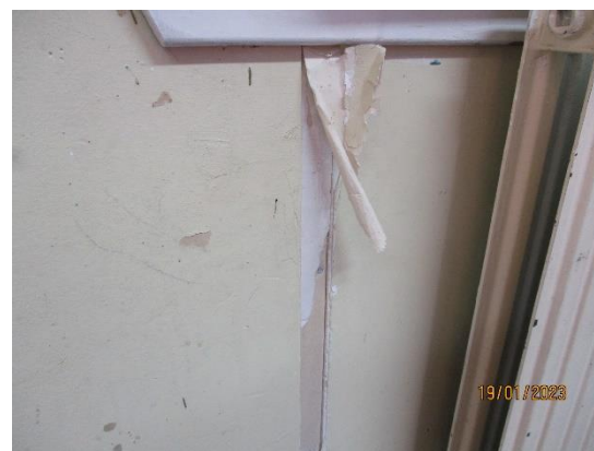
132. Failed taped joints to plasterboard
