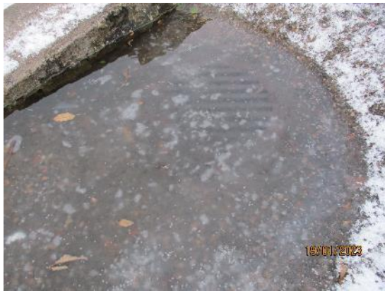
315. Blocked, flooded drainage
