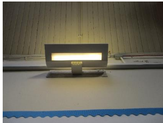
246. Lighting main school hall 1/33
