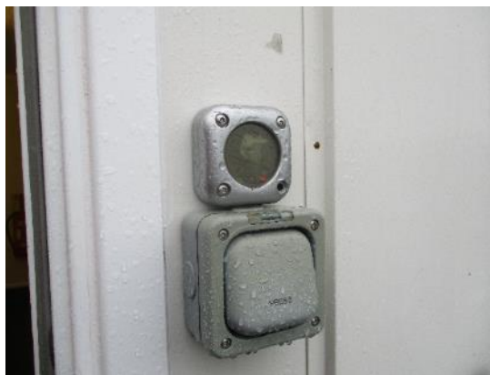
282. Door access fob reader – ASN building main entrance.
