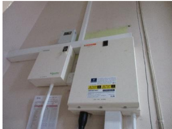
234. Distribution board – Nursery utility room GO5
