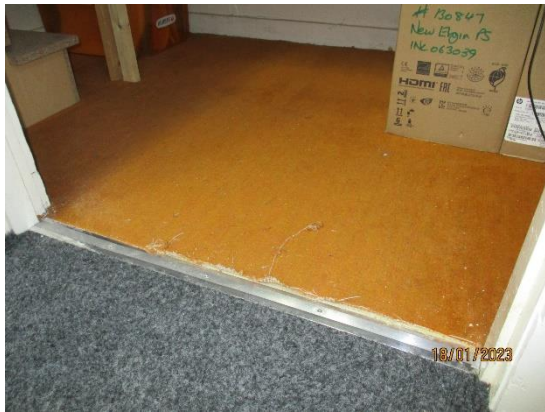
92. Damaged carpet flooring
