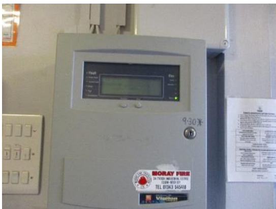
265. Fire alarm control panel main school 1/1
