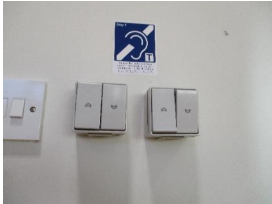
286. Electric window controls main school 1/41
