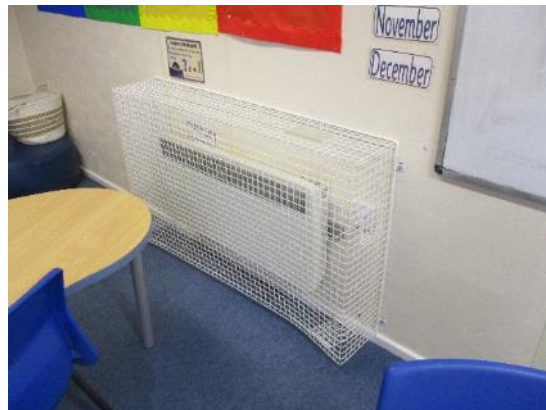
210. Electric convector with guard. ASN building.
