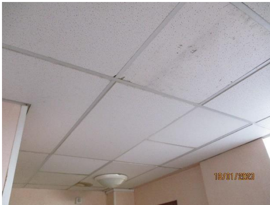
109. Suspended ceiling tiles
