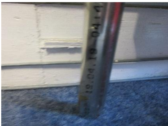
289. Pipework – new heating system.
