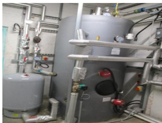
211. Calorifier – hot water storage. Main school 0/71
