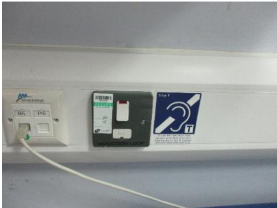
275. Induction loop system. Nursery extension
