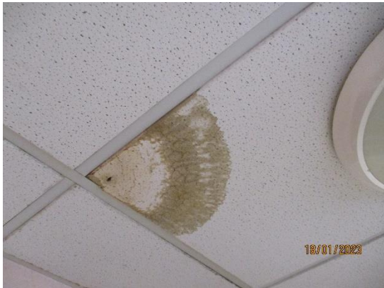
111. Watermarked ceiling tiles
