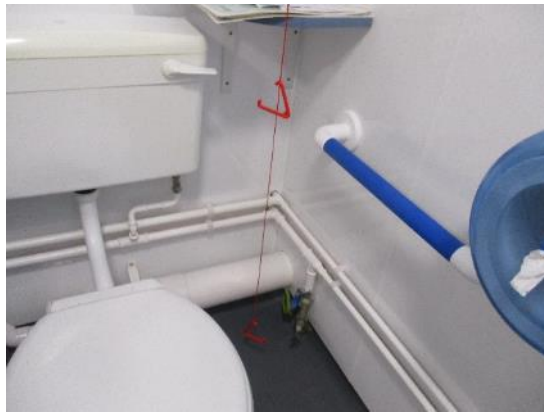
274. Disabled alarm system pull chord activation. ASN building – typical.
