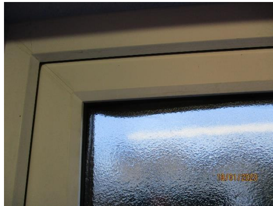
67. Glazing seals failing
