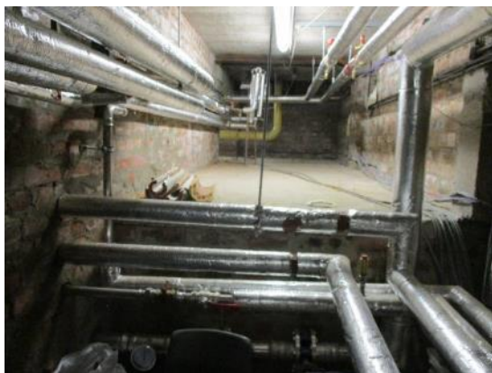
217. Pipework – hot and cold and heating main school service duct.
