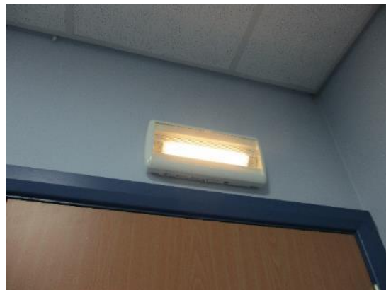
258. Emergency lighting (maintained) nursery.
