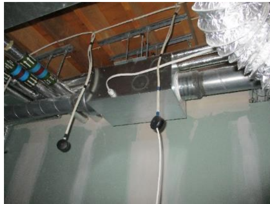
226. Heat recovery unit. Serves nursery kitchen area
