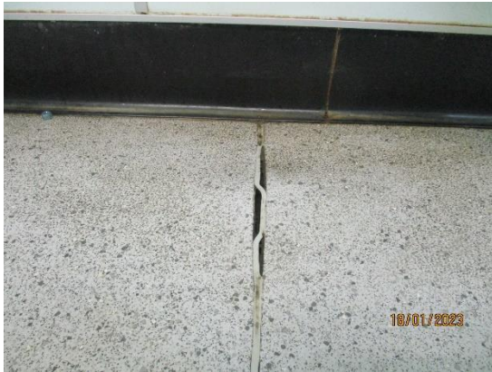
86. Open joints in vinyl flooring
