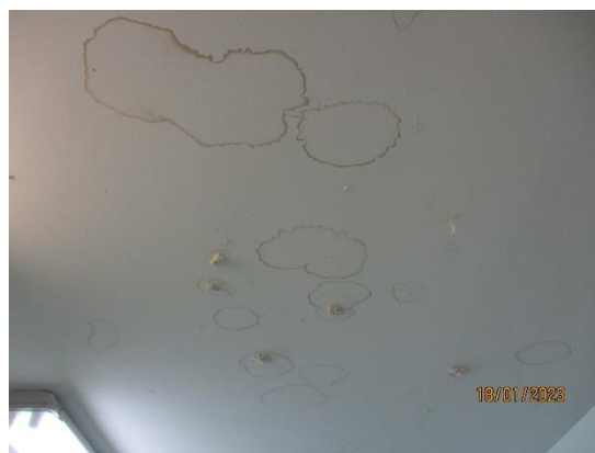
185. Water marked plaster/plasterboard ceilings
