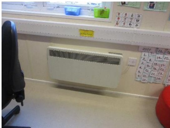
209. Electric convector – ASN building.
