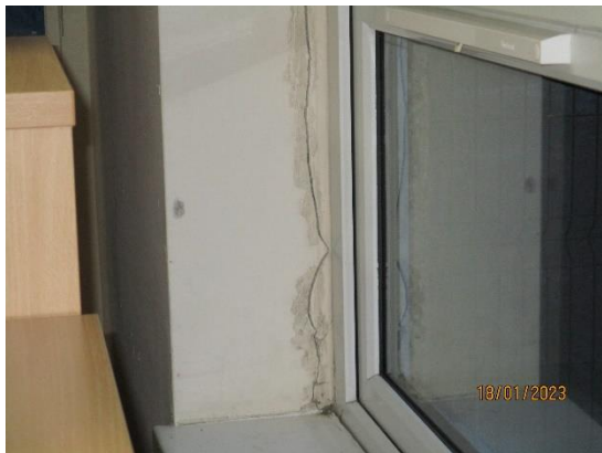
129. Cracked plaster walls
