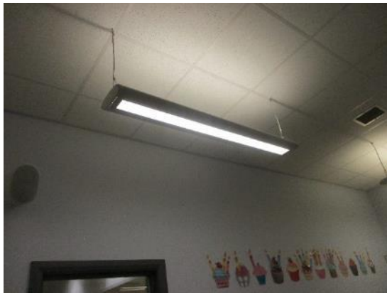
249. Lighting – nursery large room GO9
