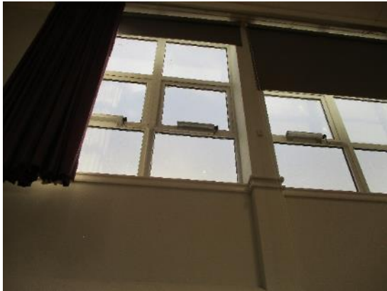
285. Electric window opening motors main school 1/41
