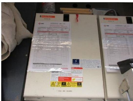
229. Distribution board main school 1/3 typical.
