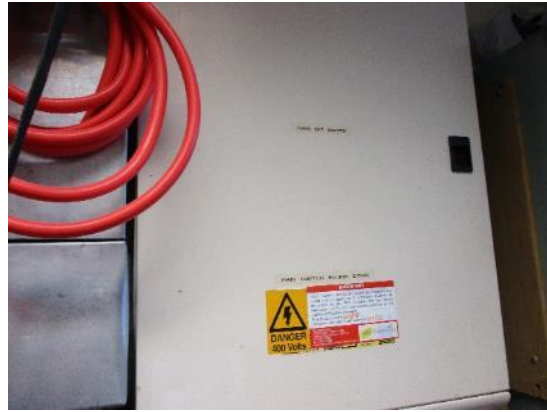
232. Distribution board main school 1/3
