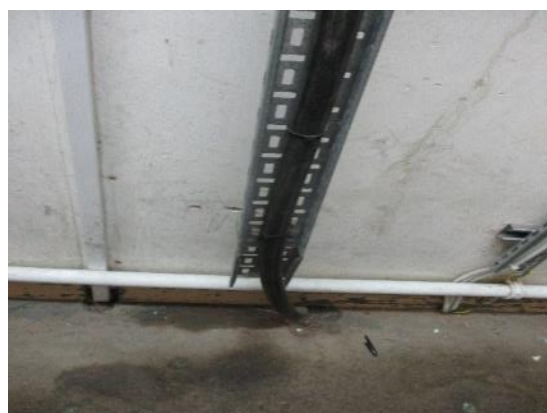
242. LV cabling – cleaners 1/39 main school
