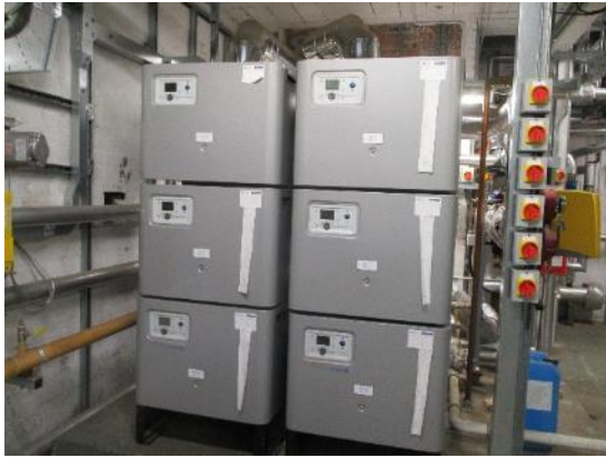
201. Boilers – Plant room 0/71
