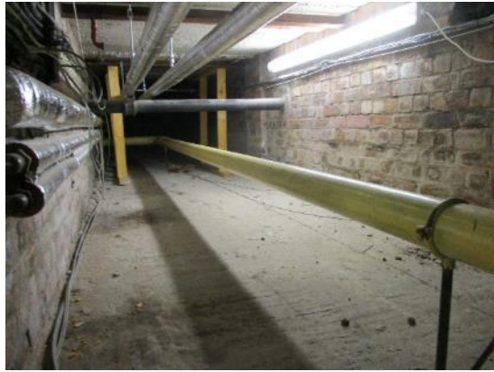
220. Gas pipe – supply to plant room under main school floor.
