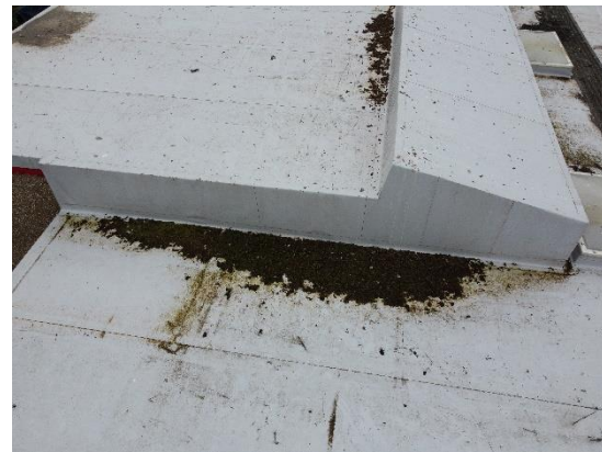
16. Debris on flat roofs
