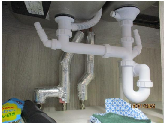
184. PVC waste pipes
