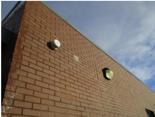
263. External lighting – nursery extension.
