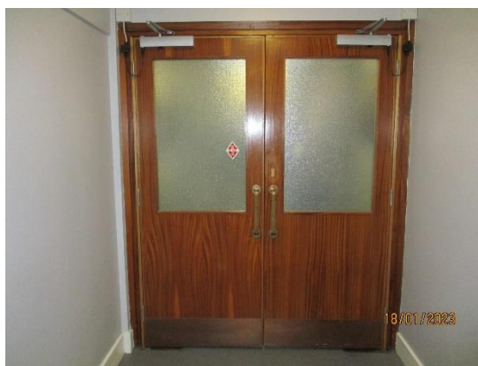
144. Double timber fire doors
