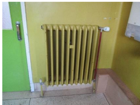
206. Radiator – cast iron. Non upgraded part of main school
