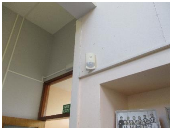
278. Intruder alarm PIR main school typical.
