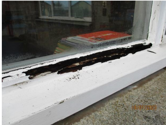
62. Rotten timber window frames
