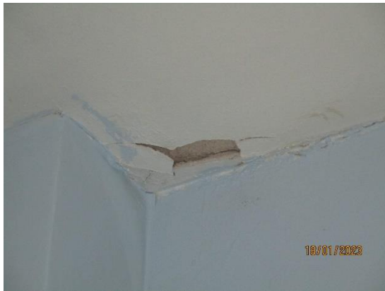
115. Cracked and spalling plaster
