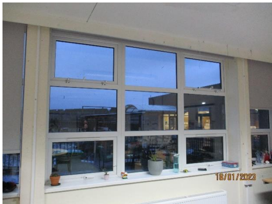
68. UPVC windows internally
