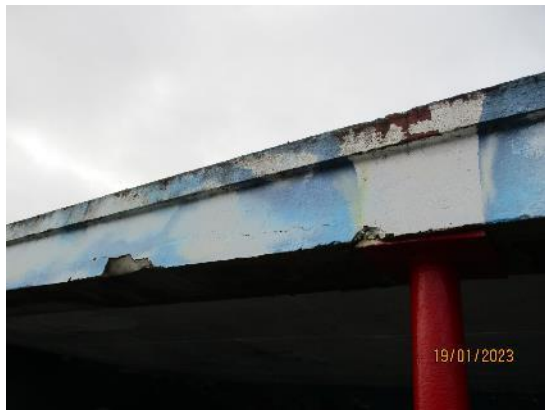
317. Spalling concrete structure
