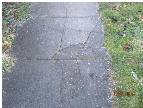
296. Damaged paving slabs
