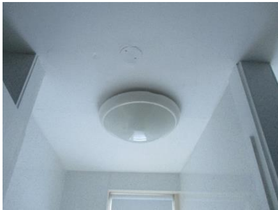
243. Lighting – main school toilets and corridors typical
