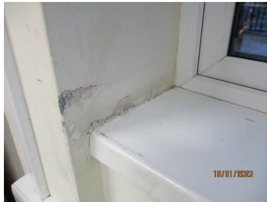
128. Damage to plastered walls
