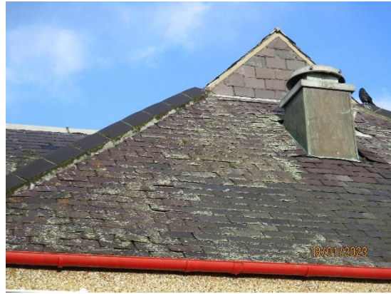
8. Slipped and broken slates
