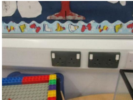
238. Sockets and dado trunking nursery typical.
