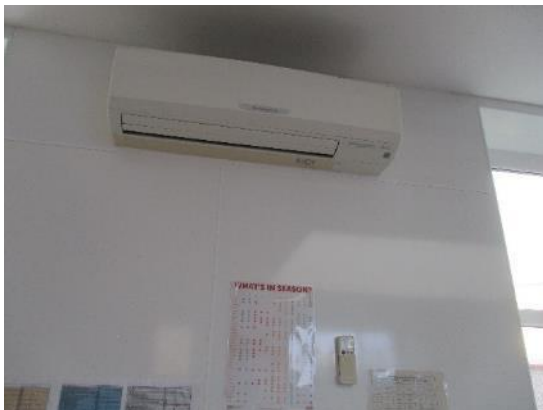
227. Air conditioning indoor unit. Main school kitchen 1/44
