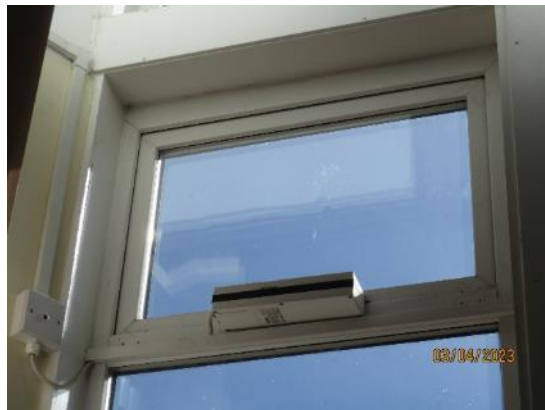
45. Electric window openers
