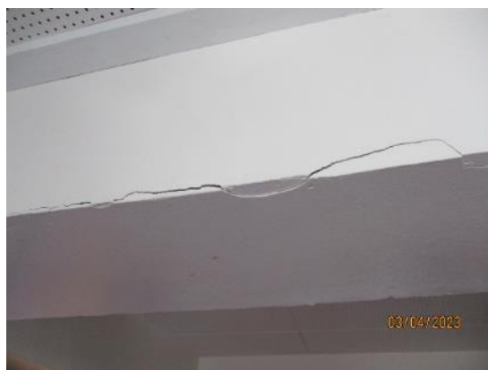
70. Cracking to concrete beams in corridors
