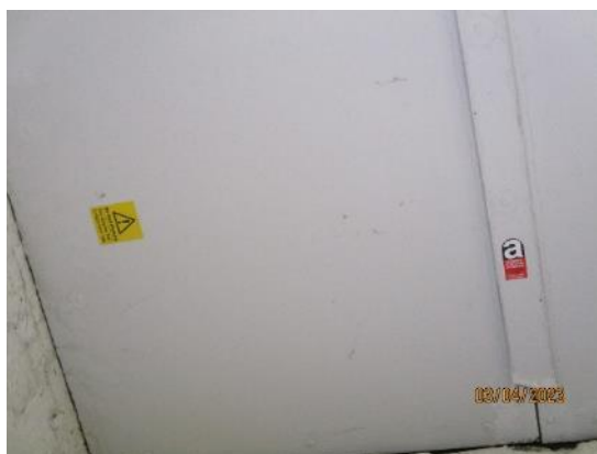
69. Labelling on ACM sheeting in the Boiler Room
