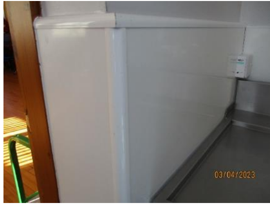
78. Wetwall in commercial kitchen
