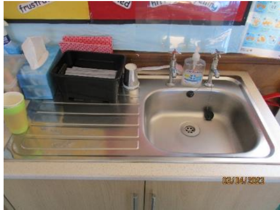
102. Stainless steel sinks in classrooms
