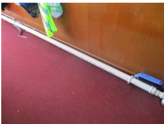
122. Pipework – heating system 1-4 class
