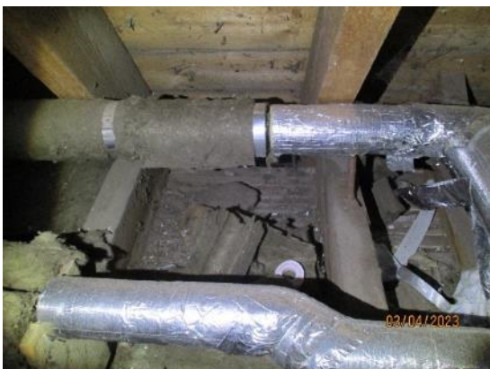
17. Insulation missing from lath & plaster ceilings
