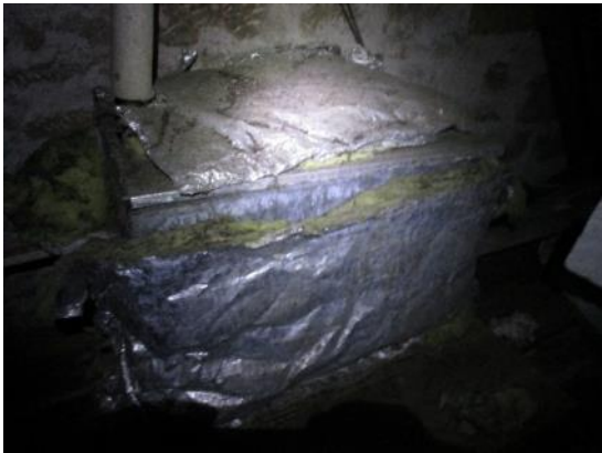
114. Heating Feed and Expansion tank. Attic above 1/5
