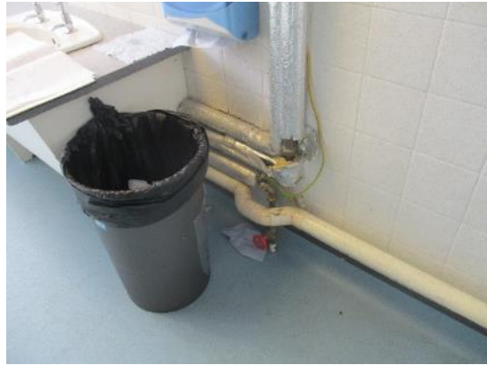
127. Pipework – hot and cold. Boys 1/5
