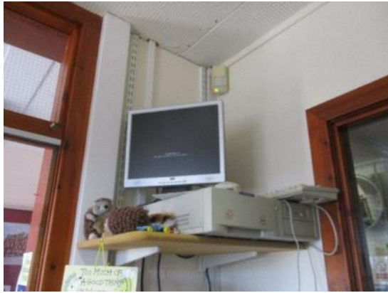
154. CCTV Monitor and processor office 1/8
