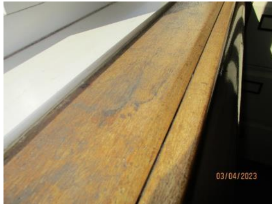
109. Timber window sills
