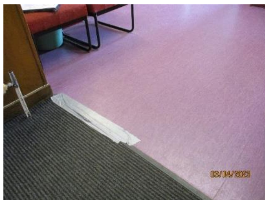
52. Isolated tape repairs
