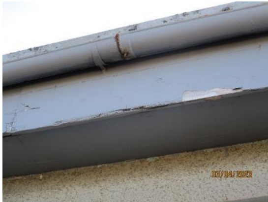
15. Early evidence of fascia timber rot
