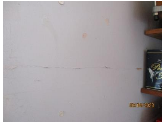
74. Hairline cracks in lath and plaster walls
