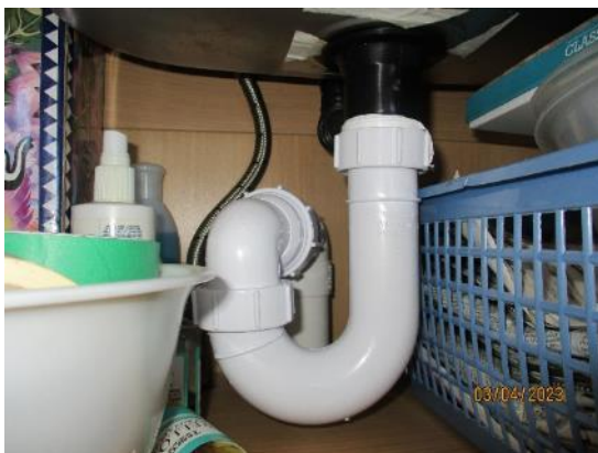
105. PVC waste pipes
