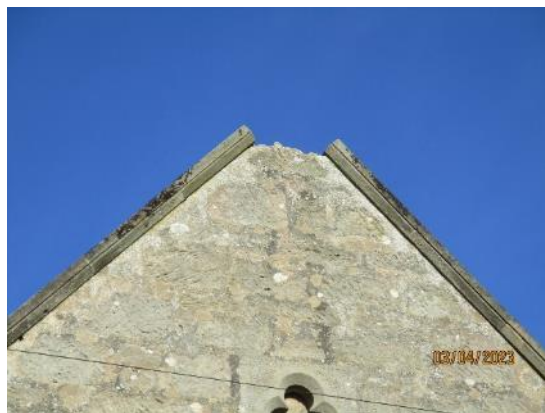
29. Missing apex stone and finial
