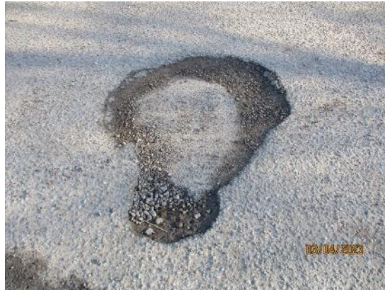
161. Potholes in tarmacadam
