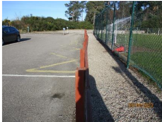
175. Some posts leaning
