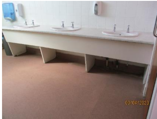
98. Basin vanity units
