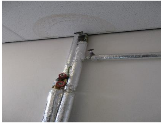
125. Pipework – Cold water Boys 1/5
