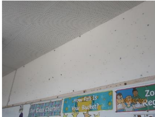
107. Marked plaster walls
