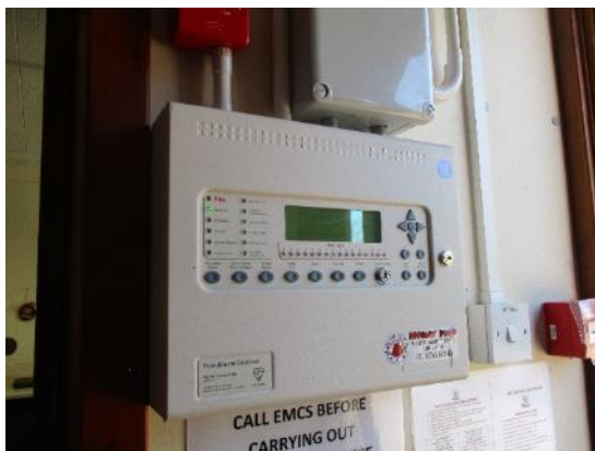
146. Fire alarm control panel entrance 1/1 lobby
