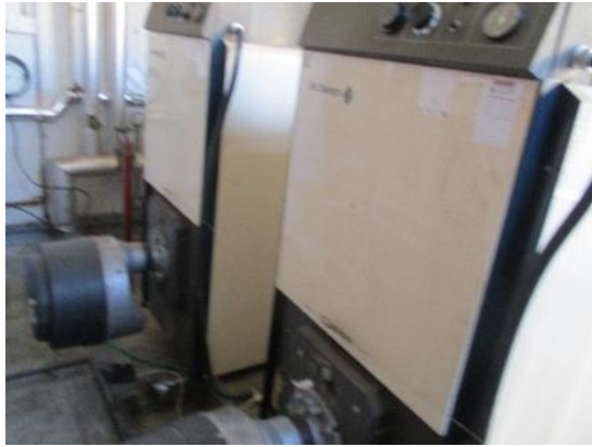
112. Oil fired boilers – Boiler house 0/14
