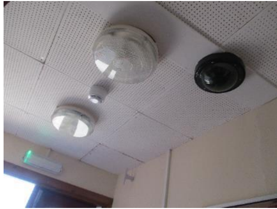
155. CCTV fixed camera 1/1 entrance lobby.
