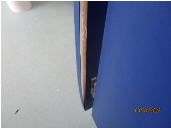
97. Loose edge trim on cubicle partition
