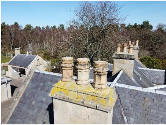
25. Chimney copes require repointing
