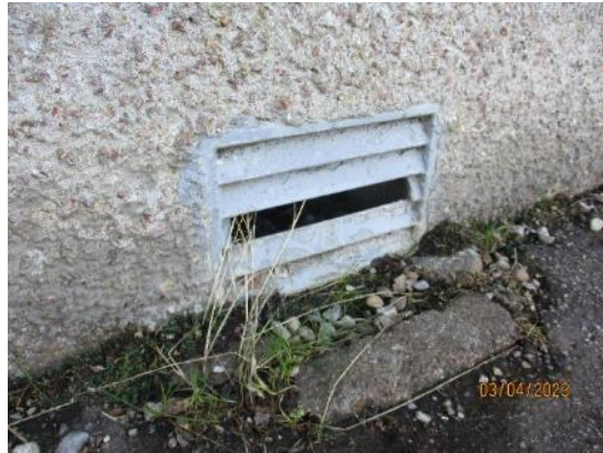
31. Broken louvre grills
