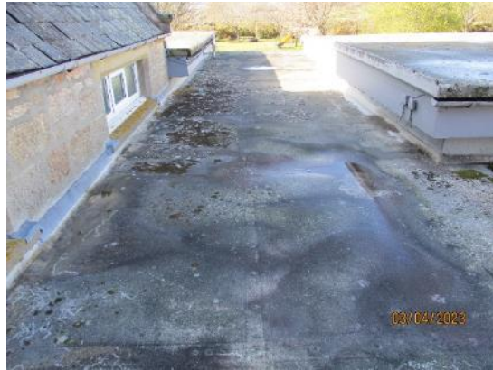
8. GRP roofs are blistered and uneven
