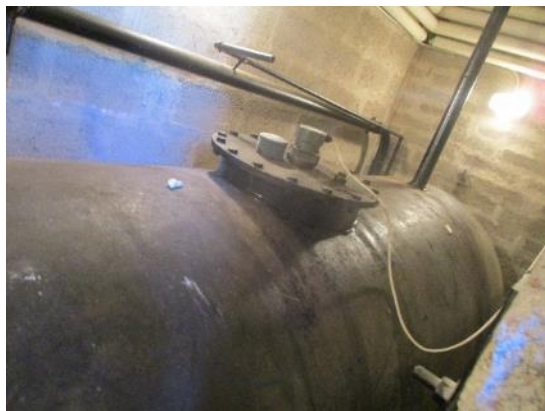
128. Oil tank in bunded room within 0/14 boiler house.
