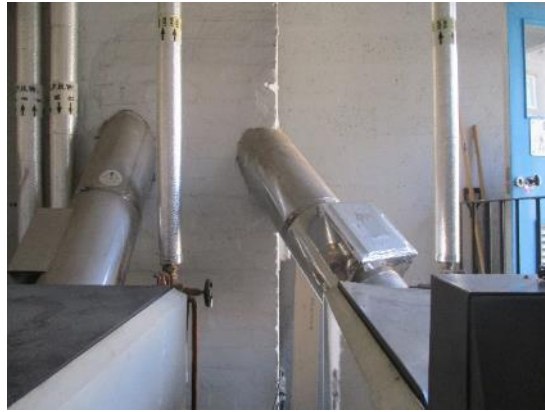
113. Boiler flues into brick chimney. Room 0/14
