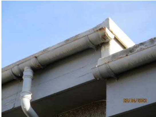
19. Leaks from gutter joints
