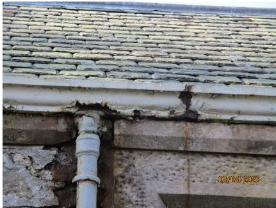
21. Cast iron ogee gutter in poor condition
