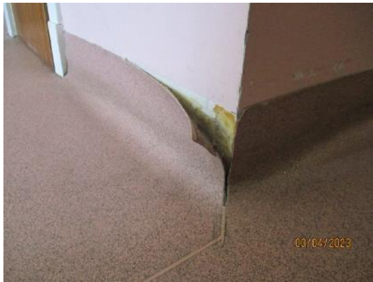
53. Coved skirting damage in Girls toilet
