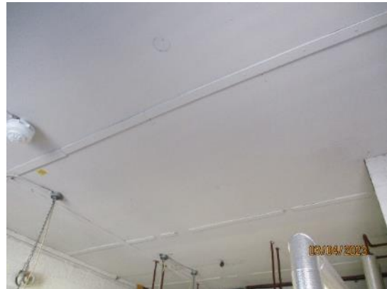
68. Sheeting with asbestos content in the Boiler Room
