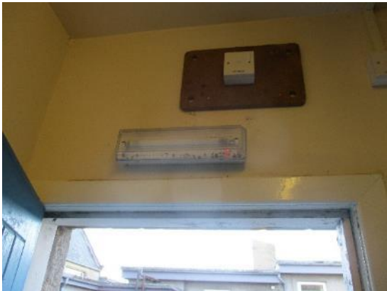
144. Emergency light 1-15a Store
