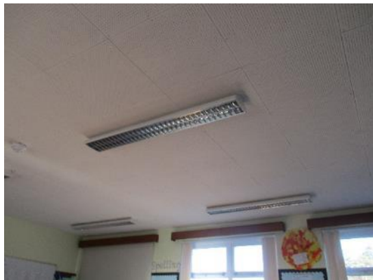
138. Lighting – Classroom typical
