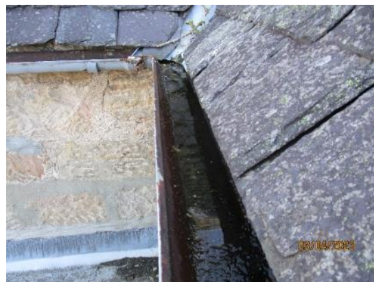
18. Cast iron gutters with some standing water
