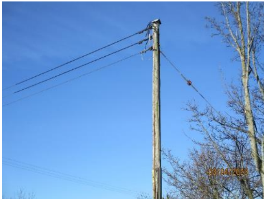
186. Timber utility pole with power lines
