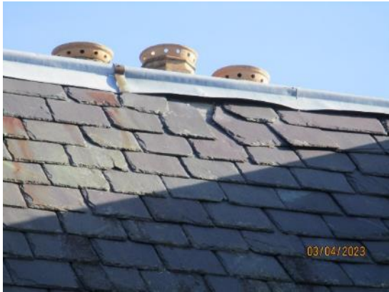
7. Isolated slate damage
