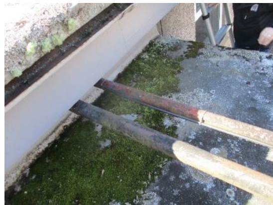
129. Oil fill and vent pipework. High level above 1/2a
