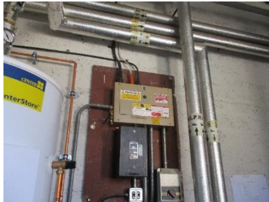
133. DB – LP2 Boiler room 0/14
