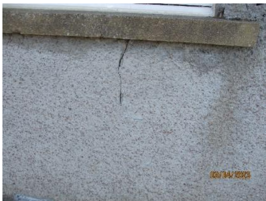
35. Vertical cracks at regular intervals
