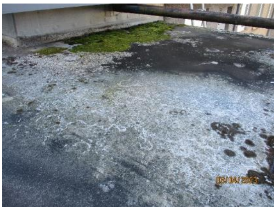
11. Vegetation and silt in sheltered areas
