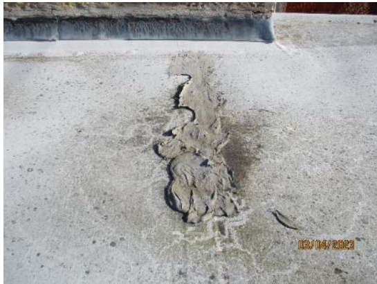
10. Evidence of previous patch repairs
