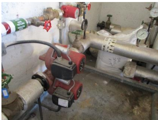
116. Pumps and Pipework – Heating system Room 0/14
