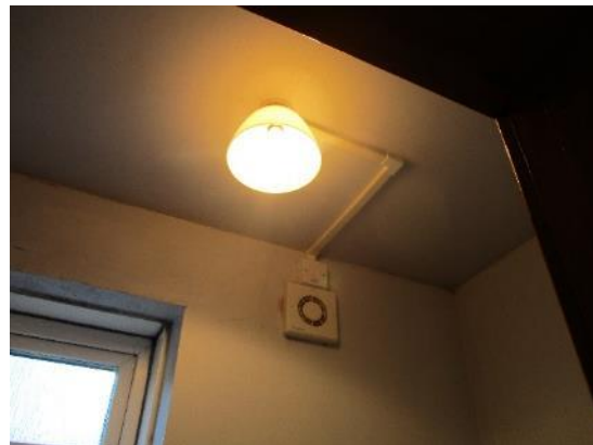
139. Lighting - stores and small rooms typical
