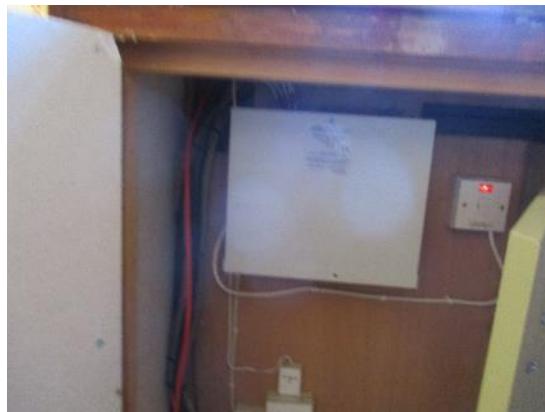
151. Intruder alarm control panel 1/2 cupboard.
