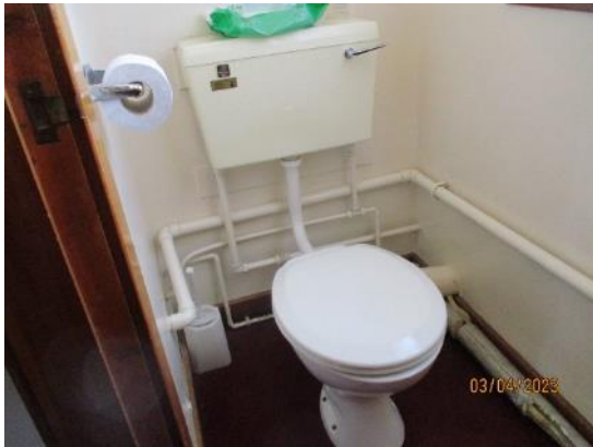
91. Staff WC with plastic cistern
