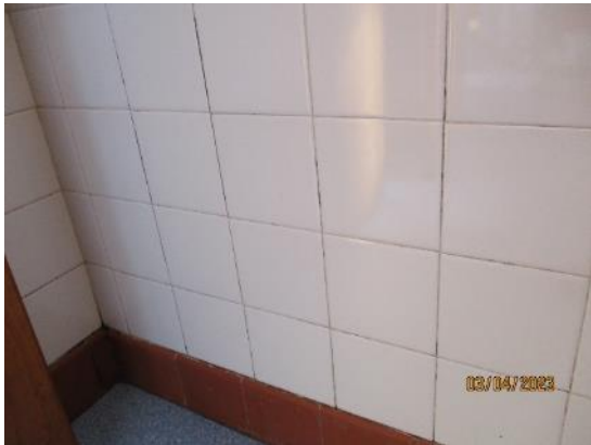
79. Ceramic tiles with soiled grouting
