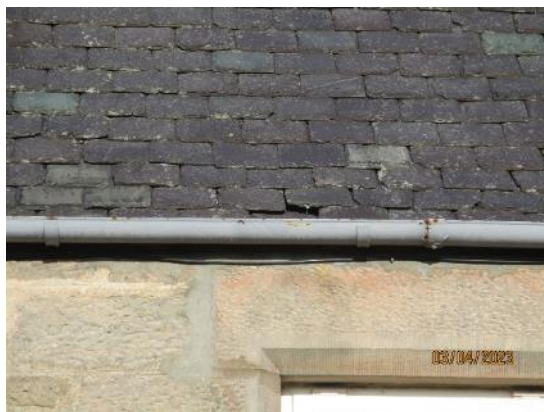
6. Isolated slate damage
