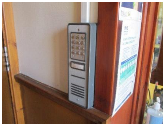
152. Door access audio and keypad 1/1 lobby.
