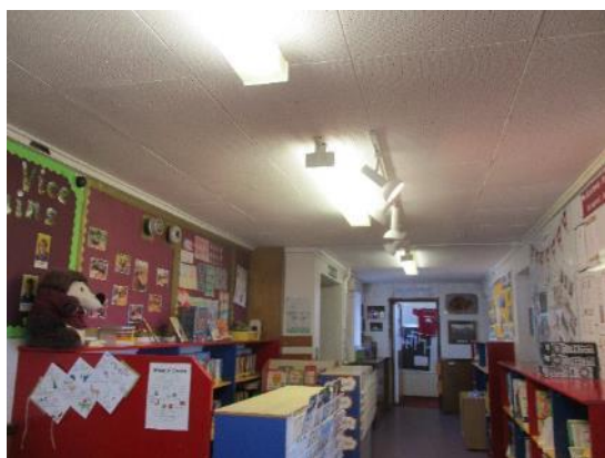
140. Lighting corridor 1/2 typical
