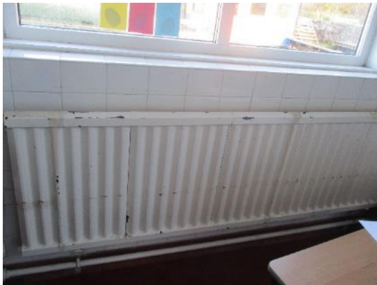
118. Radiator – Class room typical
