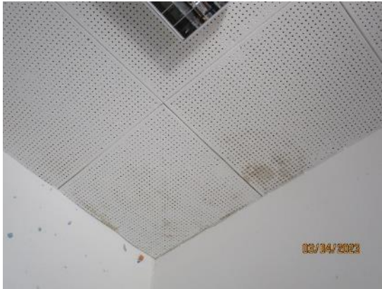
106. Water marked ceiling tiles
