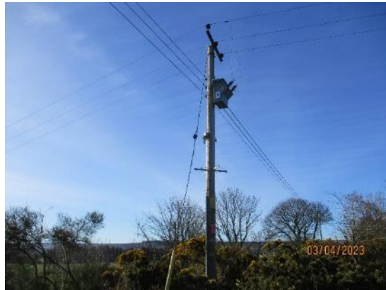
187. Timber utility pole with transformer
