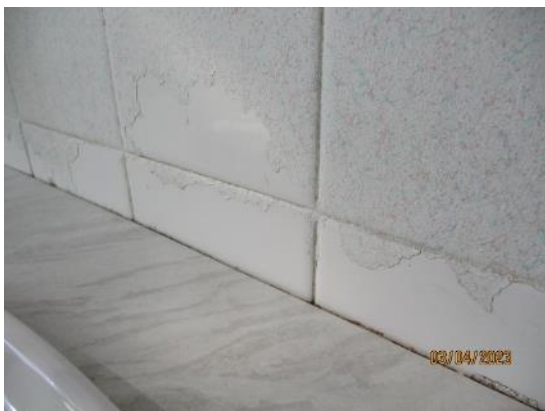
81. Ceramic tiles with paint finish peeling
