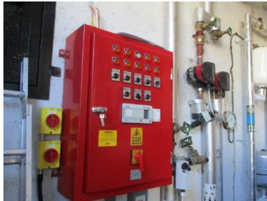
115. Heating Control Panel – room 0/14
