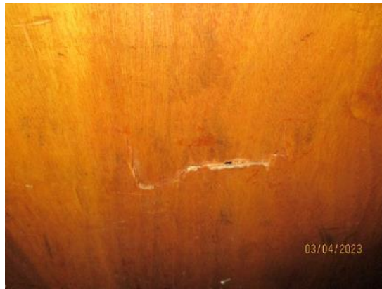
84. Surface damage to timber hollow core doors
