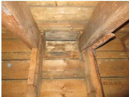
2. Isolated rot in sarking boards
