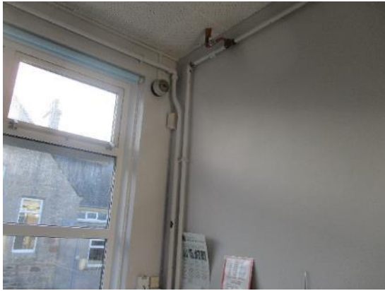
124. Pipework – hot water distribution kitchen 1/11
