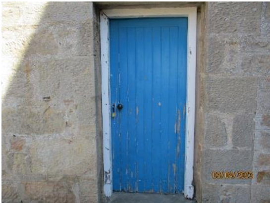
38. Rot and surface damage to timber linings of external store
