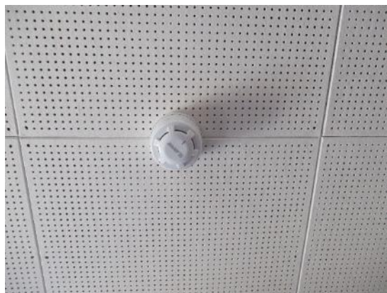
147. Smoke detector typical – wireless.
