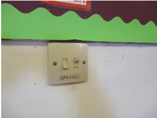
136. Light switch - typical
