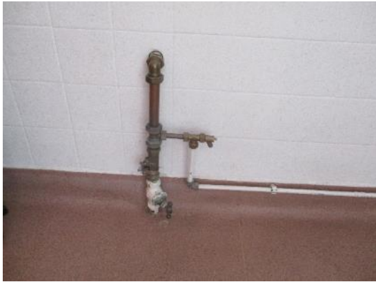
126. Pipework – cold / girls 1/6
