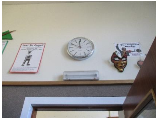
145. Emergency light HT Office 1/3
