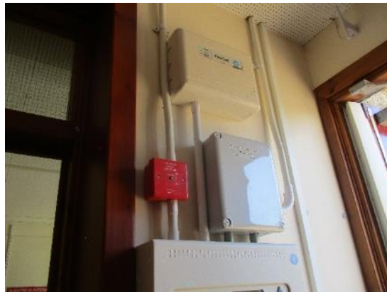
149. Fire alarm Zone hub control unit.
