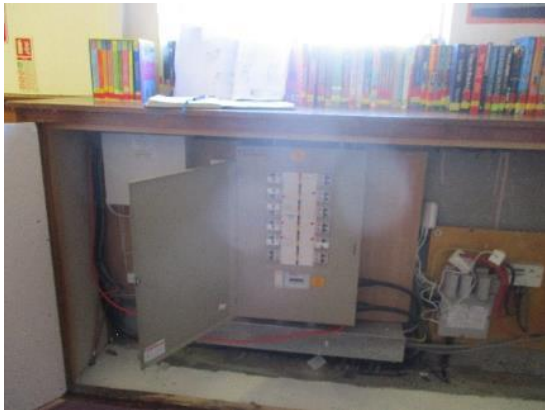
132. DB (main) Corridor 1/2 cupboard
