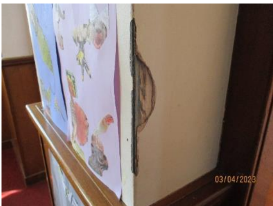
75. Isolated damage to plastered walls
