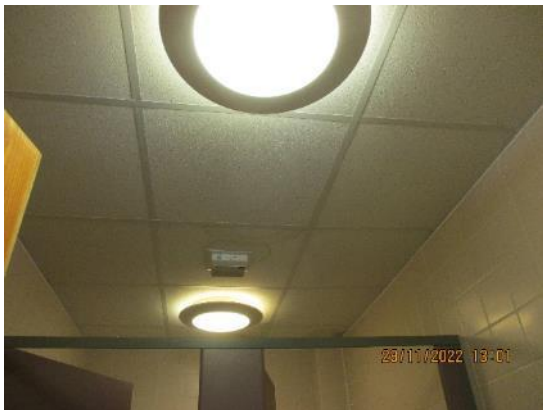
175. Lighting – toilets typical.
