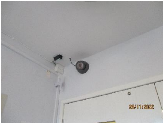
193. CCTV internal camera typical.
