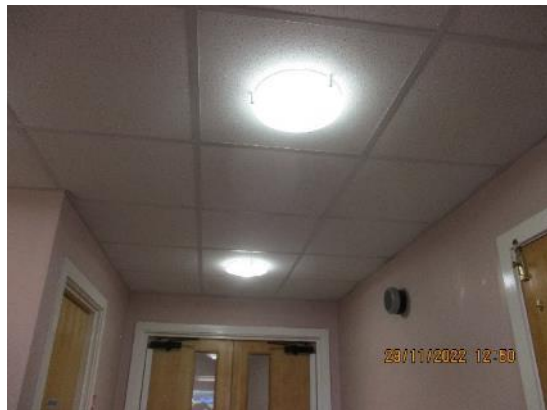
176. Lighting SEN corridor typical.
