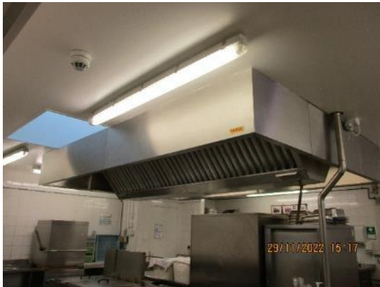
163. Extract canopy. Main kitchen.
