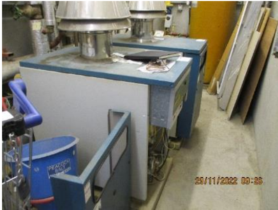
137. Boilers – SEN extension 1/54
