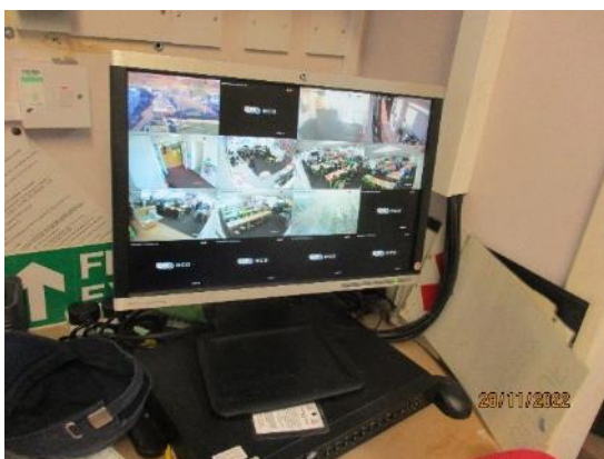
195. CCTV monitor and recorder room 1/18
