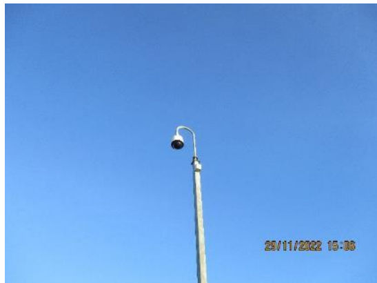
194. CCTV camera external whole site.
