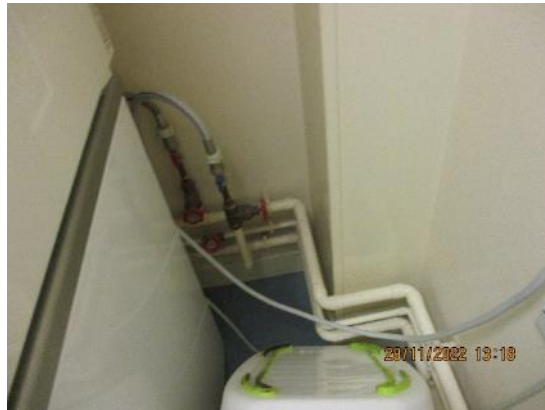
146. Pipework hot and cold. Copper – SEN laundry.
