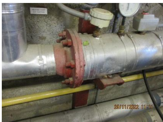
133. Heating pipework – main school 1/54
