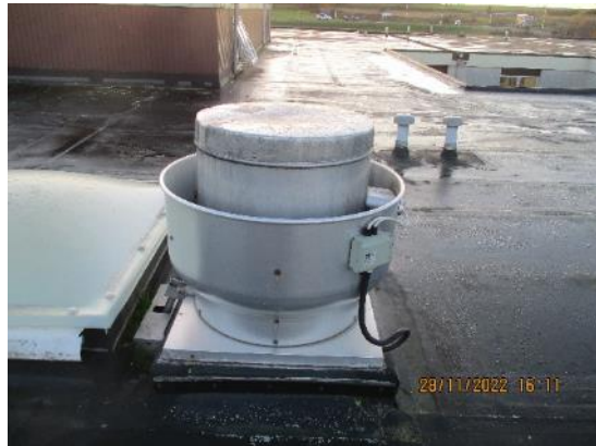
164. Extract fan. Kitchen canopy – roof mounted.
