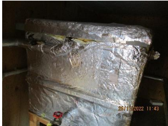
144. Cold water storage tank. SEN zone roof housing.
