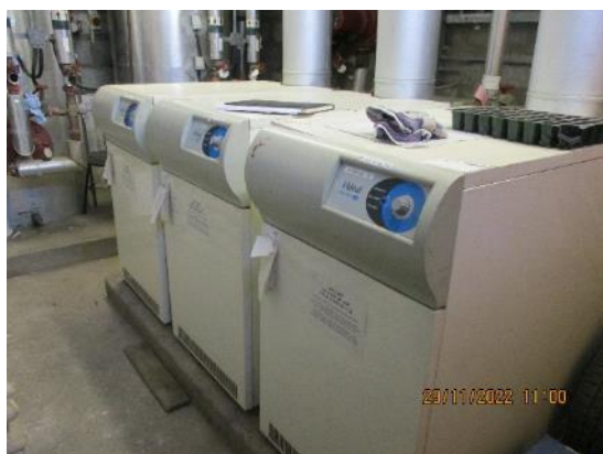
131. Gas boilers – main school plant room 1/54
