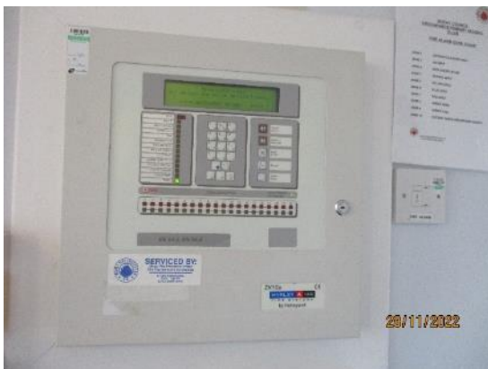
183. Fire alarm control panel – main school entrance.
