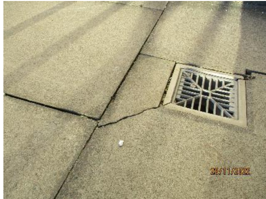
216. Broken paving slabs
