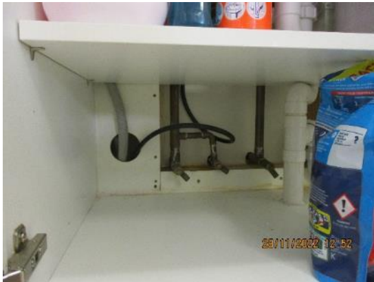
145. Pipework – hot and cold copper SEN kitchen
