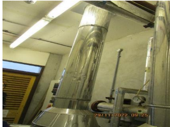
138. Flue – boilers SEN extension 1/54
