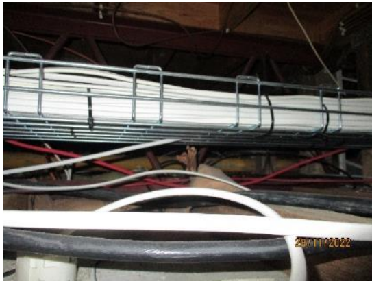
169. General wiring main school ceiling void.
