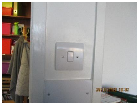
178. Light switch manual control typical.
