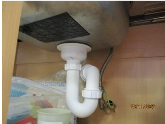
123. UPVC waste pipes
