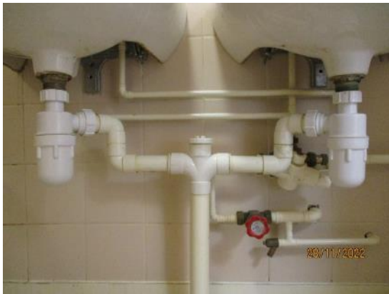
110. PVC waste pipes
