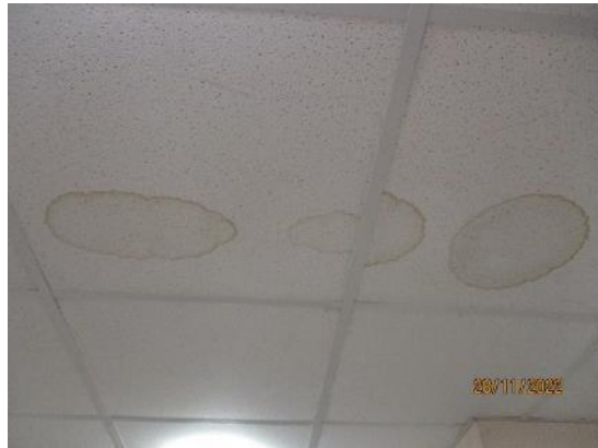
73. Water marked ceiling tiles
