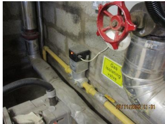
156. Gas pipework and solenoid control valve to kitchen. Located in 1/55.
