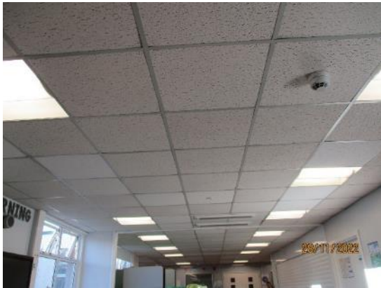
72. Suspended ceiling tiles
