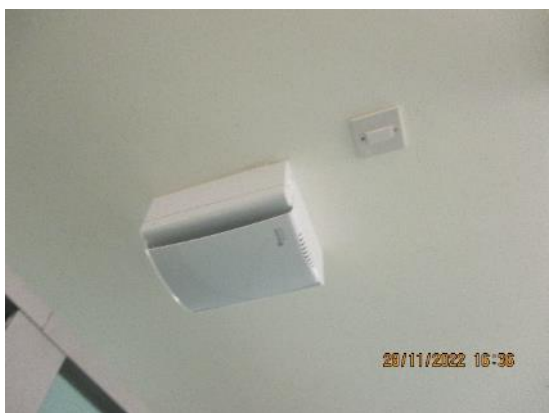
160. Extract fan. Boys toilets 1/38
