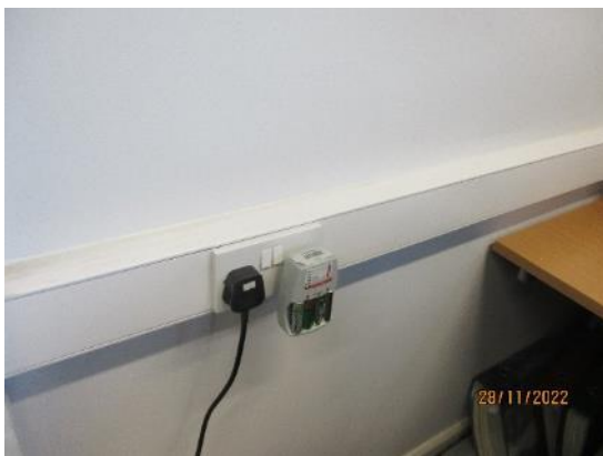
171. Sockets and dado trunking – main school typical.
