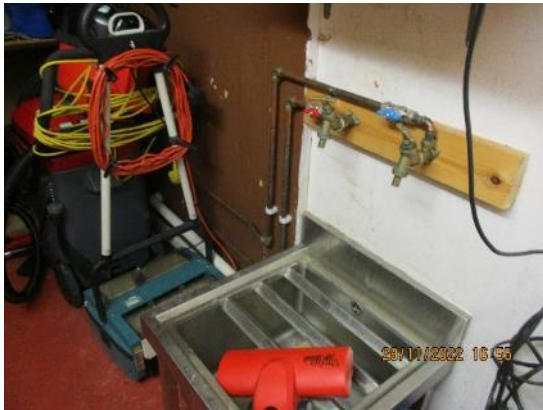
151. Pipework – hot and cold. Main school Cleaners store 1/23.
