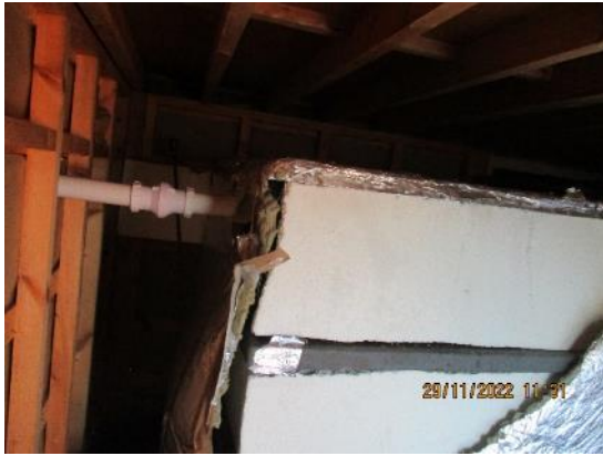
149. Cold water tank 4. Main school roof housing.
