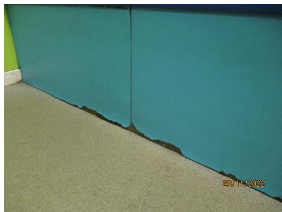
115. Damaged base units
