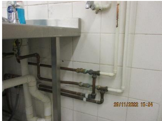
152. Pipework – hot and cold. Main school kitchen.
