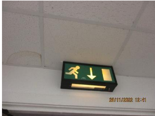
180. Emergency exit maintained light. Typical.
