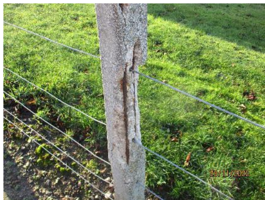
220. Damaged concrete posts
