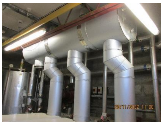
134. Boiler flues – main plant room 1/55
