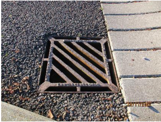
233. Car perk drainage
