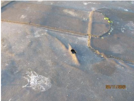
7. Holes in surface
