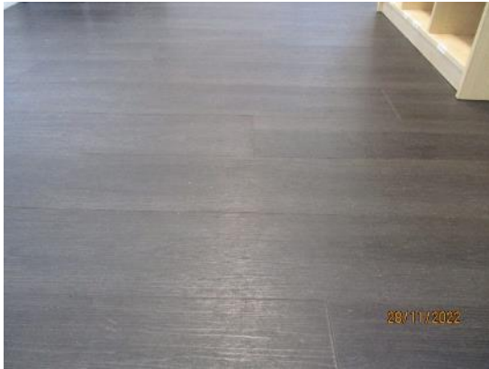
70. Laminate flooring (Reception)
