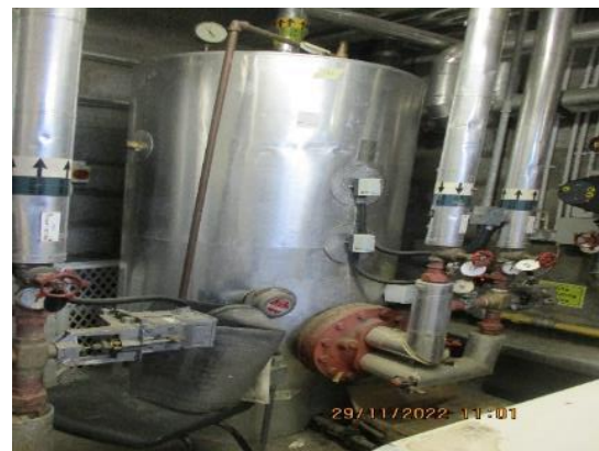
148. Hot water calorifier 2. Kitchen. Main school 1/55
