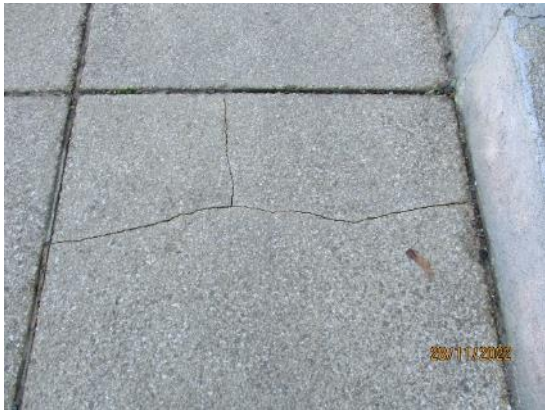
61. Broken paving slabs
