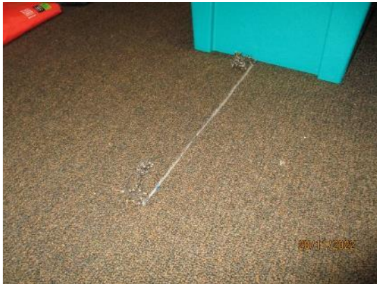
66. Damage to carpets
