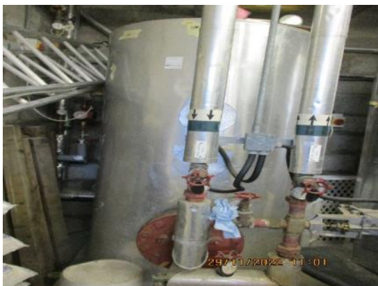
147. Hot water calorifier 1 – main school 1/55
