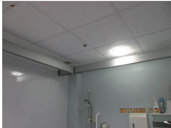
200. Hoist system traction rail – SEN girls toilets.
