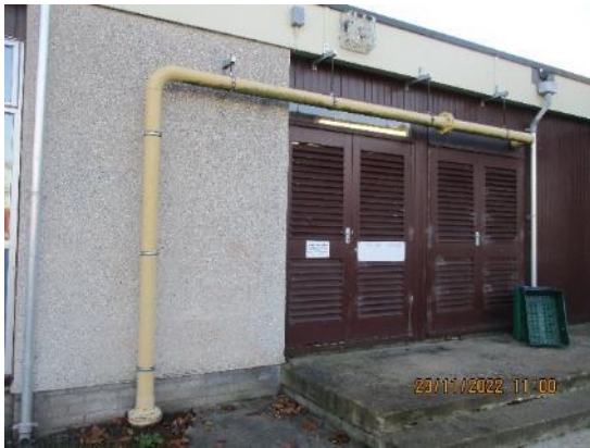
155. Gas pipe entry to main plant room 1/55
