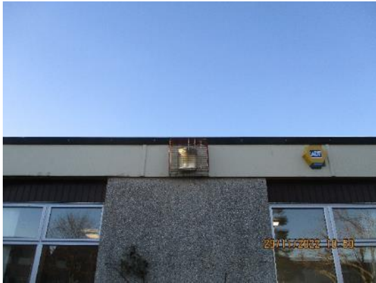
179. External building lighting. Typical
