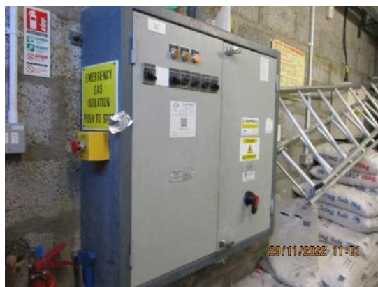
132. Heating control panel main school 1/55
