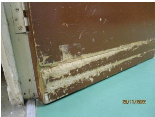
97. Damage to timber doors
