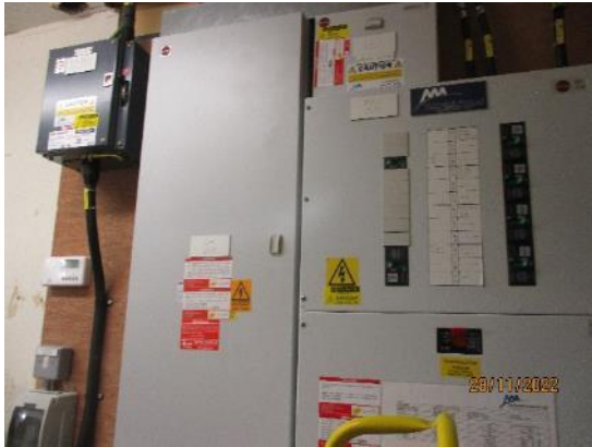
167. Distribution boards and switchgear 1/19
