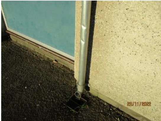
25. Minor surface damage
