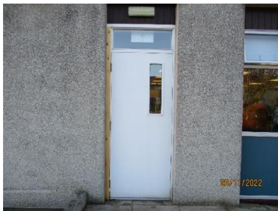
34. Timber fire exit doors
