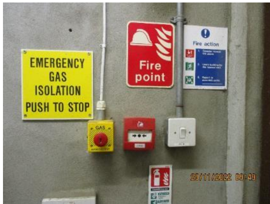
157. Gas safety stop button. Plant room 1/54
