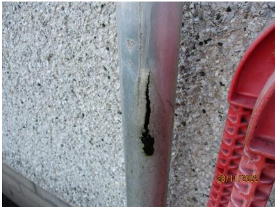
27. Split in aluminium downpipe
