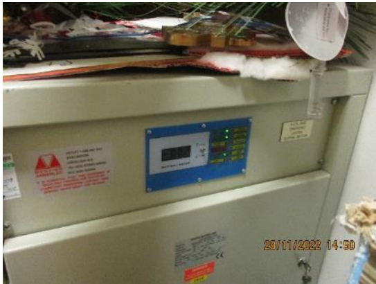
181. Emergency lighting central battery – extension 1/41
