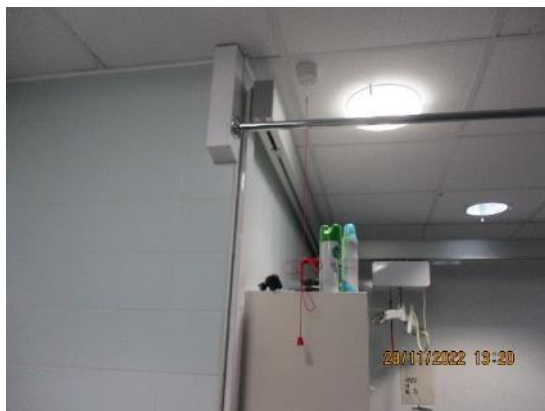
189. Intercall disabled alarm system. Pull chord SEN girls toilets.
