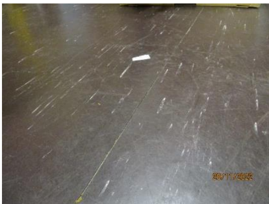
68. Sheet vinyl – open joints
