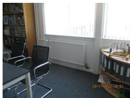
135. Radiator – steel panel. Main school 1/5
