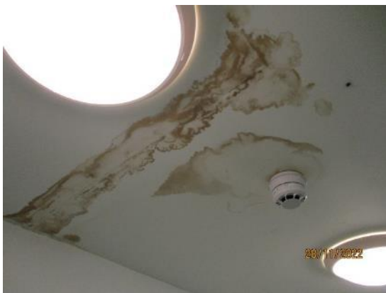
80. Water marked Plasterboard ceilings
