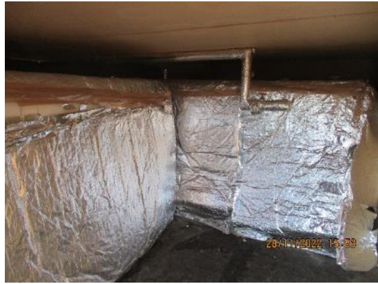
150. Cold water tanks 1+2. Main school. Roof housing.
