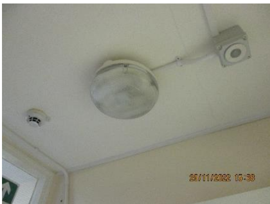
177. Lighting and PIR main kitchen stores typical.
