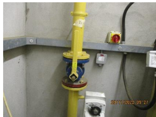
142. Gas isolation valve – SEN plant room 1-54
