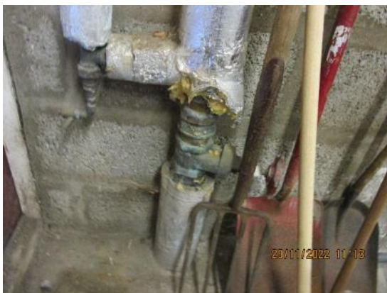
153. Pipework. Cold water mains entry to plant room 1/55
