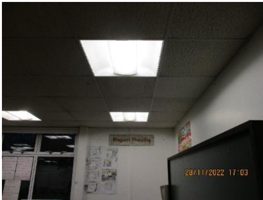
173. Lighting – classroom typical.
