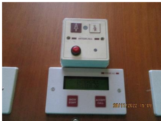
190. Intercall disabled alarm system panels typical throughout SEN extension.
