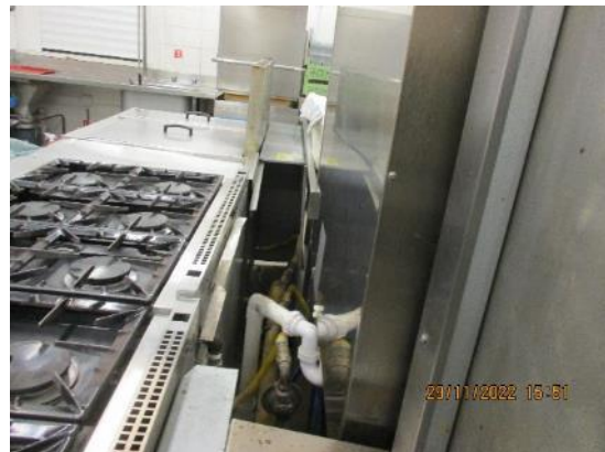
158. Gas range and pipework. Main kitchen.
