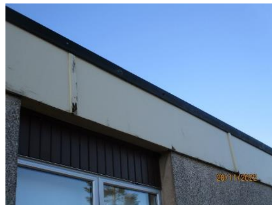
18. Rot in plywood fascia boards
