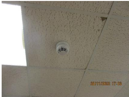
186. Fire detector head typical throughout.
