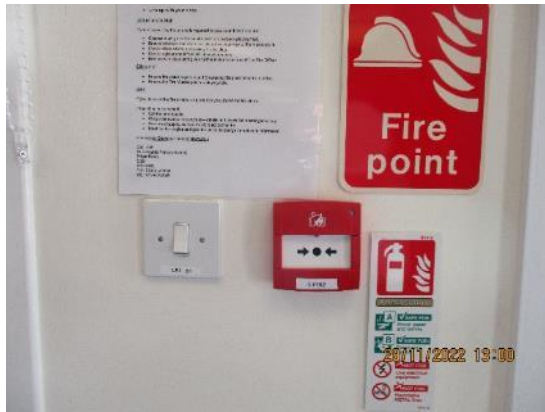
185. Fire alarm call point 1-46 SEN zone.
