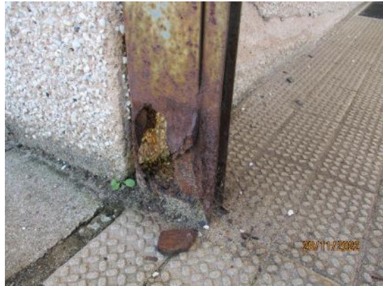
37. Extensive corrosion of steel guide rails
