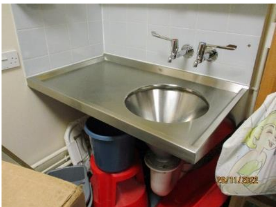
121. Stainless steel sluice (Laundry)
