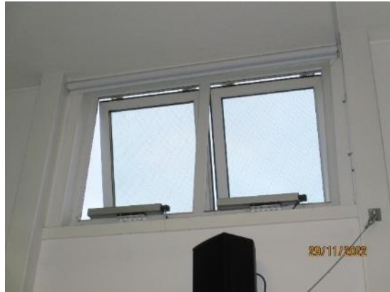
49. Electrically operated UPVC windows
