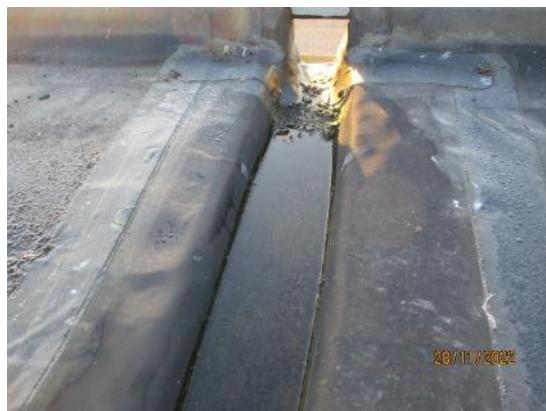
12. Box gutters blocked
