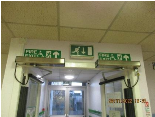
191. Automatic electric operated doors. 1/36a
