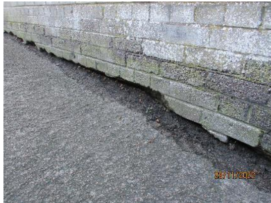
230. Damaged brick wall to rear ramp
