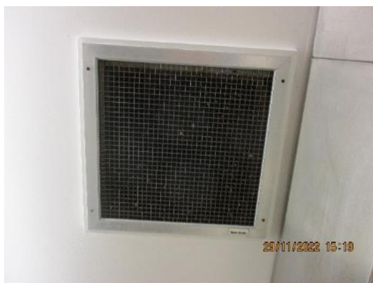
159. Extract fan. Dishwasher steam – main kitchen.
