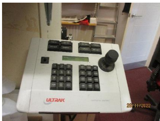
196. CCTV system user controls 1/18
