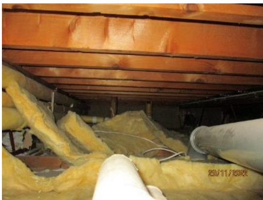
17. Thin, inadequate insulation
