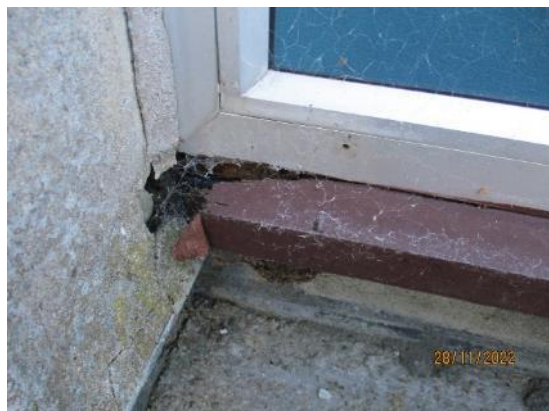
47. Rot in timber sills
