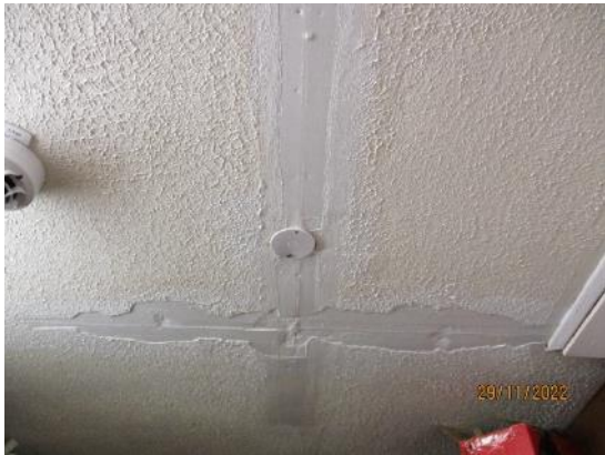
78. Damage to textured ceiling finish
