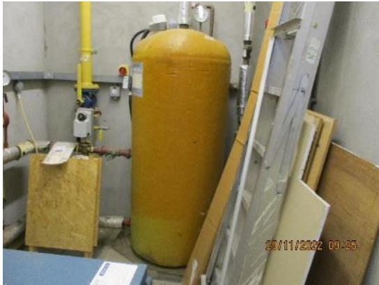
143. Hot water calorifier – SEN plant room 1/54
