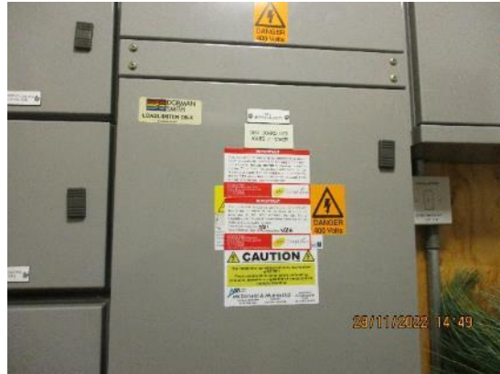
168. Distribution boards 1/41 SEN
