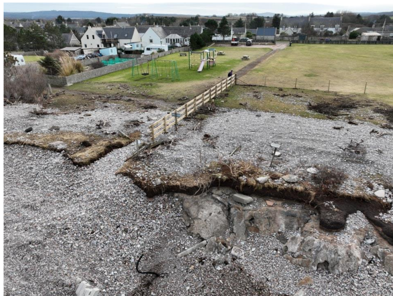
Figure 2 Erosion at Kingston Beach
