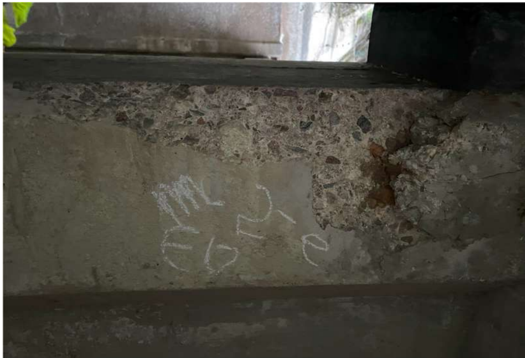
Photograph 80: Beam 5 – Beam 6, east pier, west face, concrete spalling with staining
