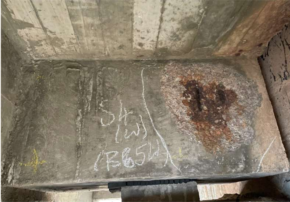
Photograph 51: Beam 5 (north facing), half joint west, spalling with exposed rebar
