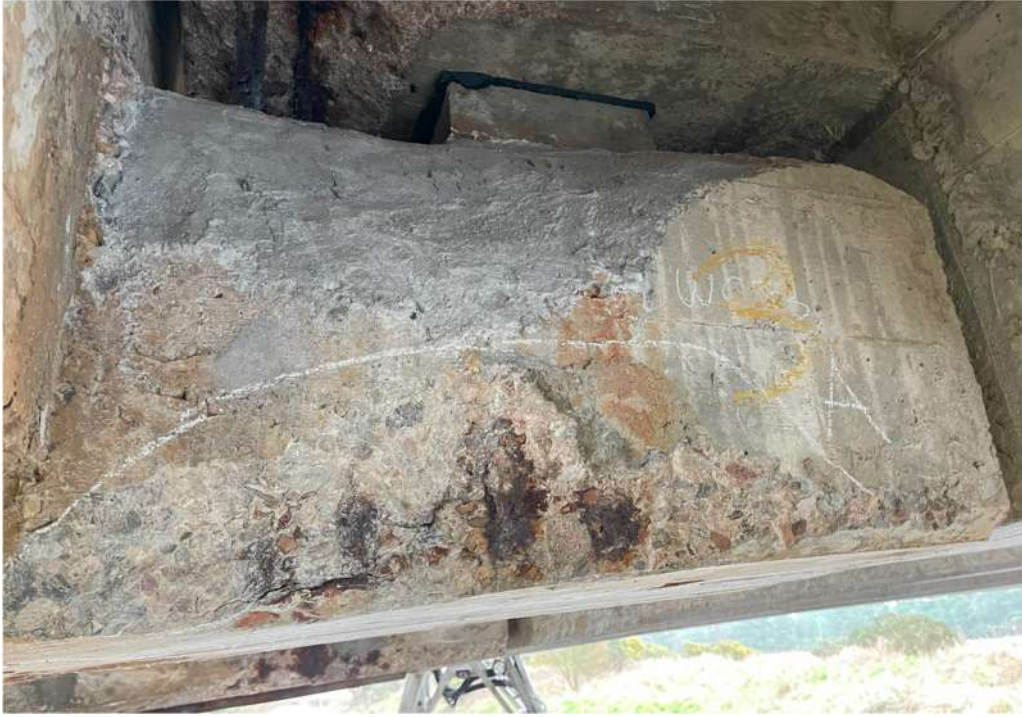
Photograph 47: Beam 3 (south facing), half joint west, spalling and exposed reinforcement, evidence of previous repair
