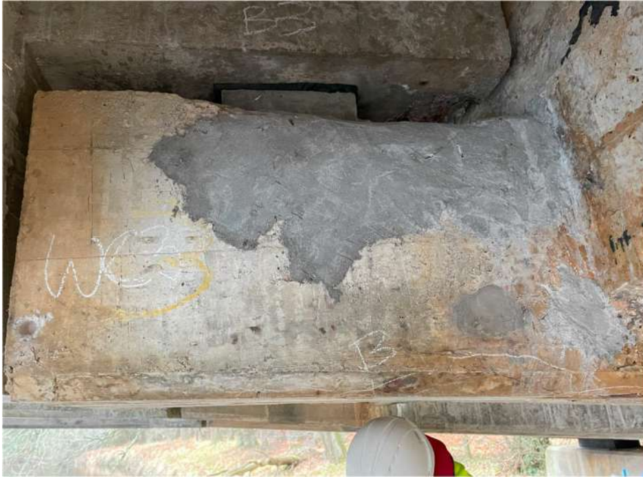
Photograph 45: Beam 3 (north facing), half joint west, crack with hairline cracks in same area
