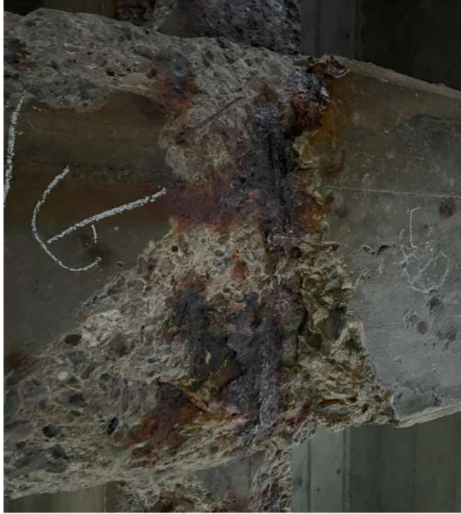
Photograph 29: Beam 5, cantilever span east, spall between crossbeams
