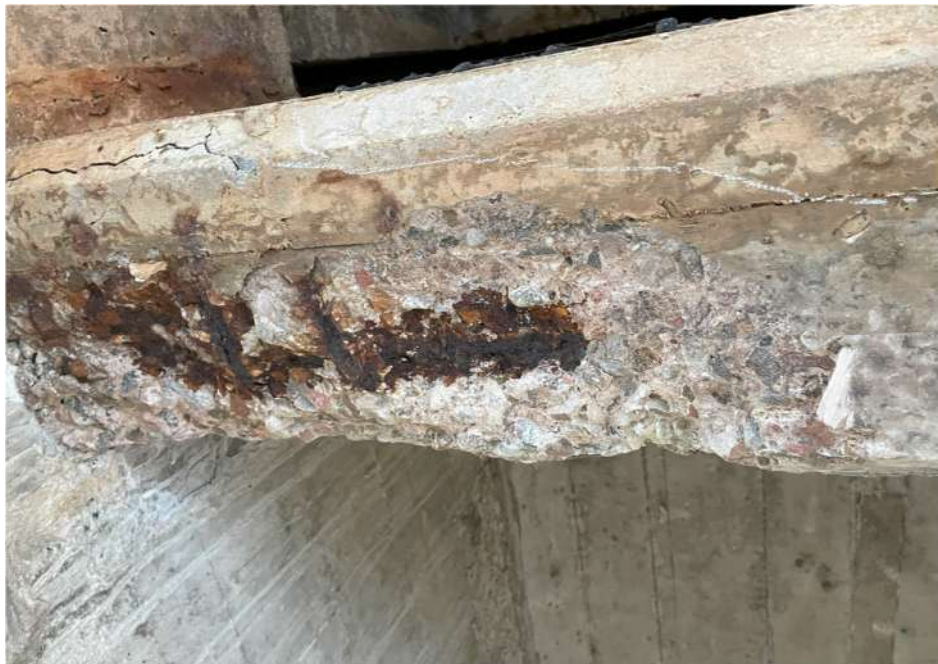
Photograph 18: Beam 3 – Beam 4, cantilever span west, cross beam, full width spall with exposed reinforcement
