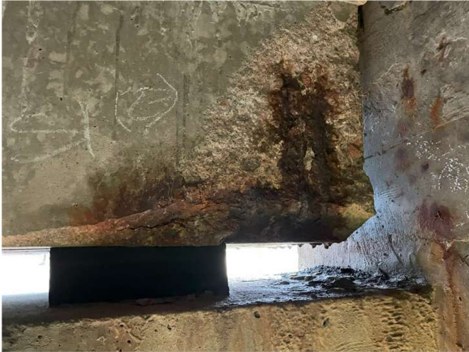
Photograph 57: Beam 1 (south facing), half joint east, spalling with exposed and corroded reinforcement
