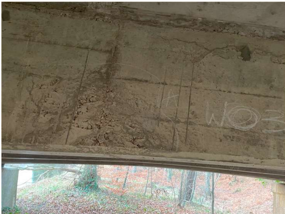
Photograph 38: Beam 3, outer span west, honeycombing on side face
