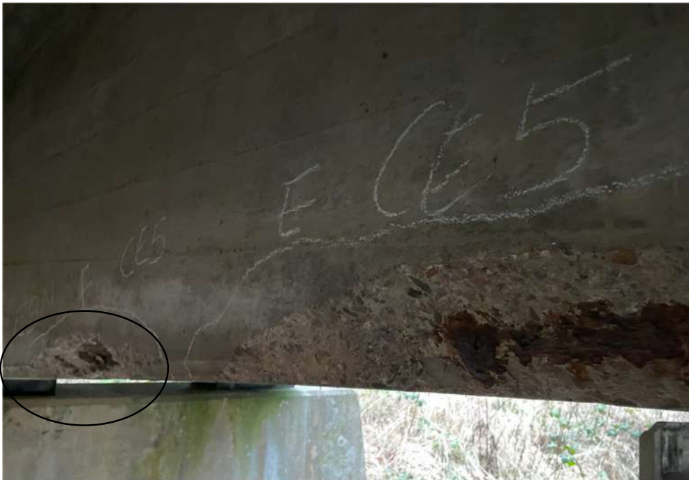
Photograph 28: Beam 5, cantilever span east, spall reinforcement exposed and corroded
