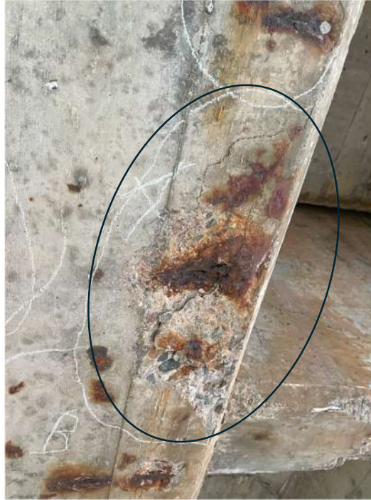
Photograph 5: Beam 2, cantilever span west, cracking and staining on bottom face
