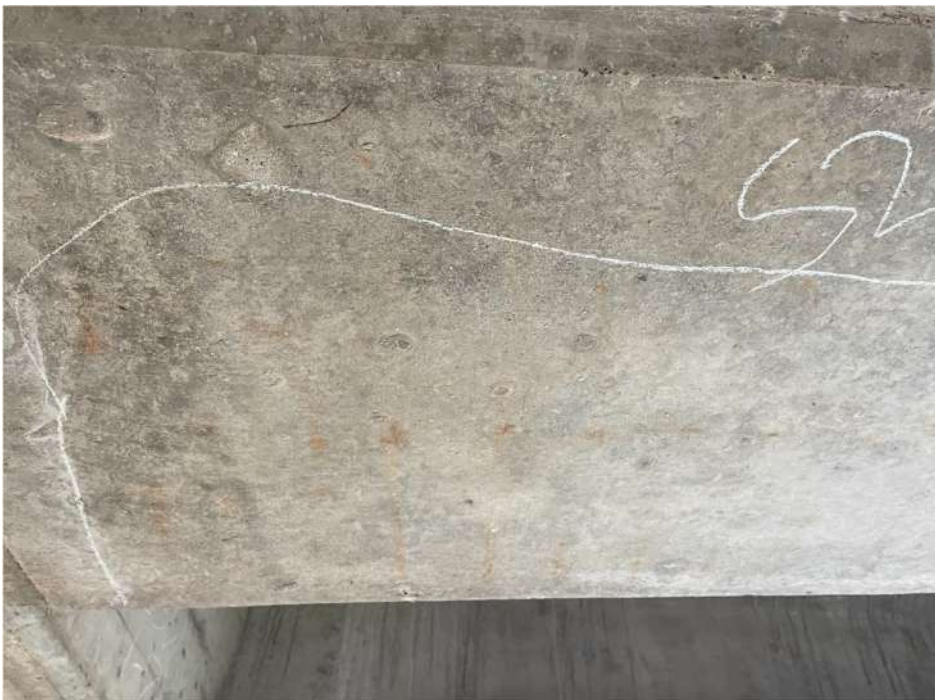
Photograph 2: Beam 2 soffit, suspended span, rebar staining
