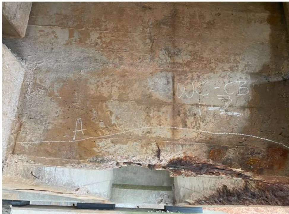
Photograph 16: Beam 1 – Beam 2, cantilever span west, cross beam, full width spall with exposed reinforcement
