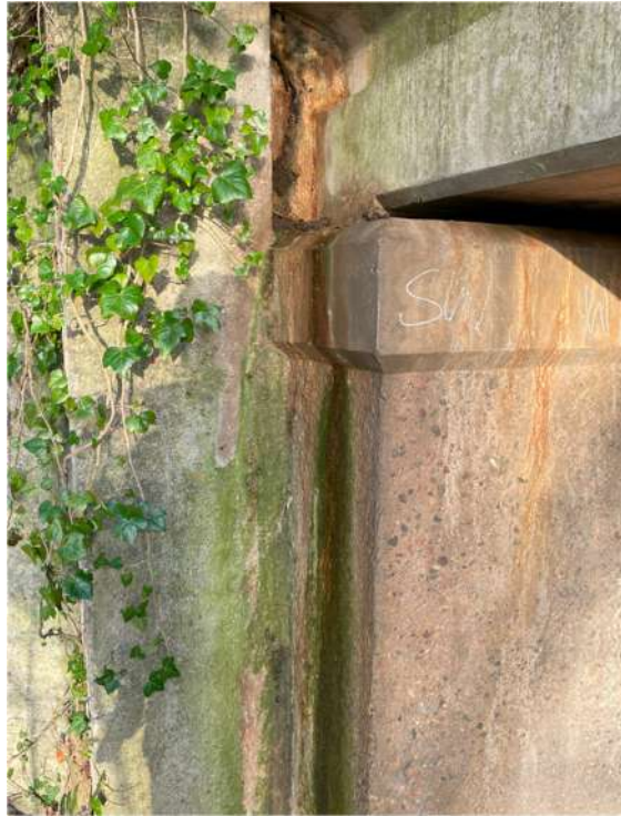
Photograph 81: Abutment corners, east and west abutment, staining and seepage, residue build up
