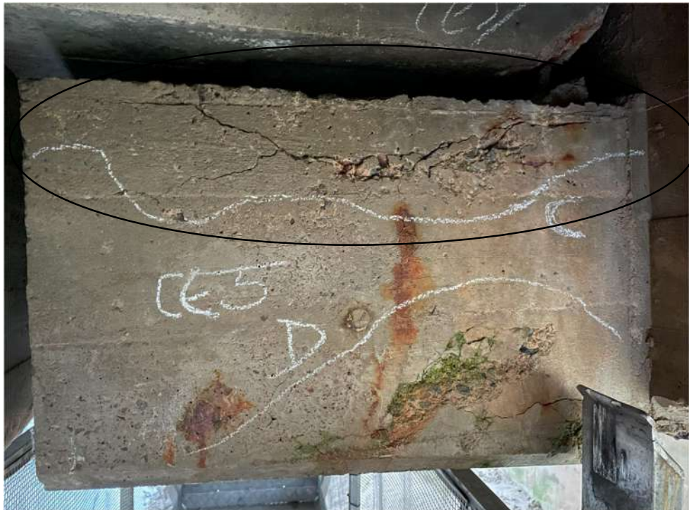
Photograph 70: Beam 5 (south facing), half joint east, crack below top edge, bursting
