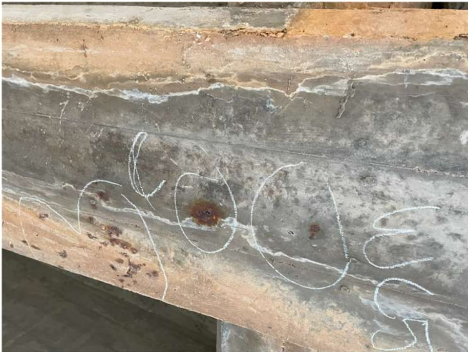
Photograph 14: Beam 5, cantilever span west, spotted corrosion marks
