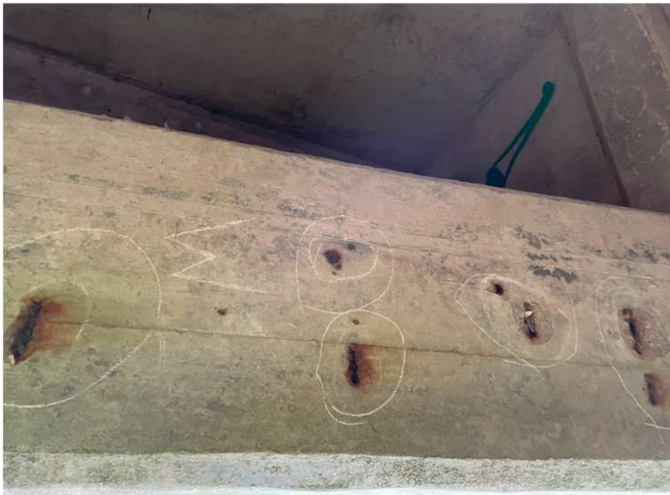
Photograph 36: Beam 1, outer span west, small areas of spalling
