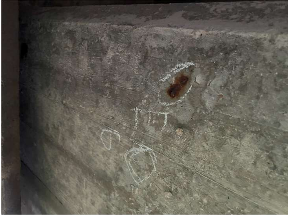
Photograph 39: Beam 6, outer span east, small spalls
