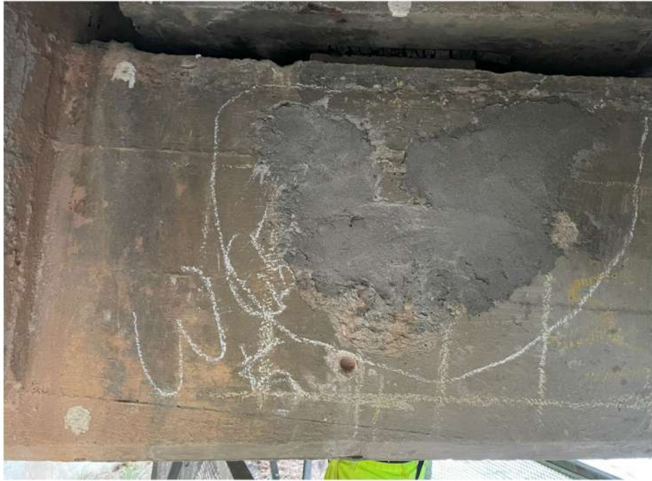
Photograph 53: Beam 5 (south facing), half joint west, previous repair with new hairline crack going into patch
