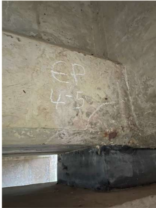
Photograph 79: Beam 4 – Beam 5, east pier, west face, hairline crack with corrosion staining
