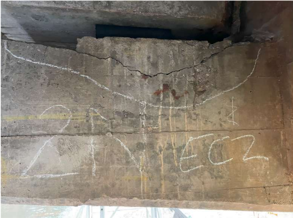
Photograph 61: Beam 2 (south facing), half joint east, spalling concrete indicated by cracking, bursting off corner
