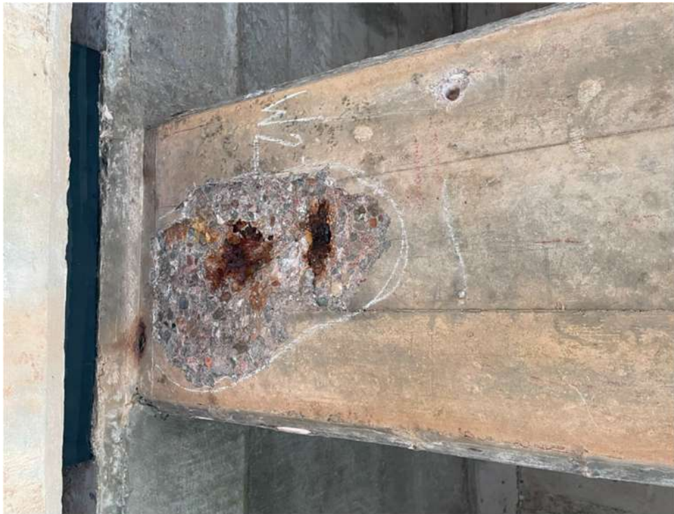
Photograph 10: Beam 2, cantilever span west, exposed and corroded reinforcement
