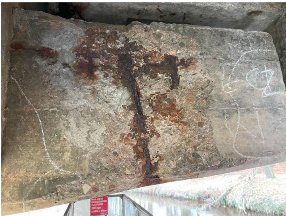
Photograph 62: Beam 2 (north facing), half joint east, exposed and severely corroded reinforcement
