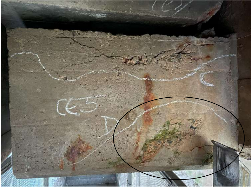
Photograph 71: Beam 5 (south facing), half joint east, spalling with cracking present
