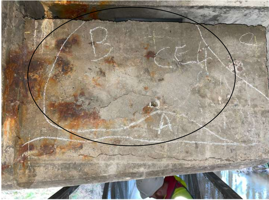
Photograph 67: Beam 4 (north facing), half joint east, delaminated face of beam
