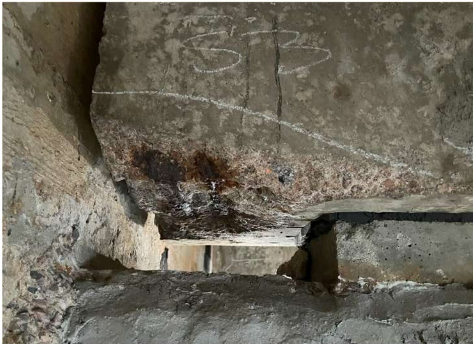
Photograph 46: Beam 3 (south facing), half joint west, spalled corner with exposed reinforcement
