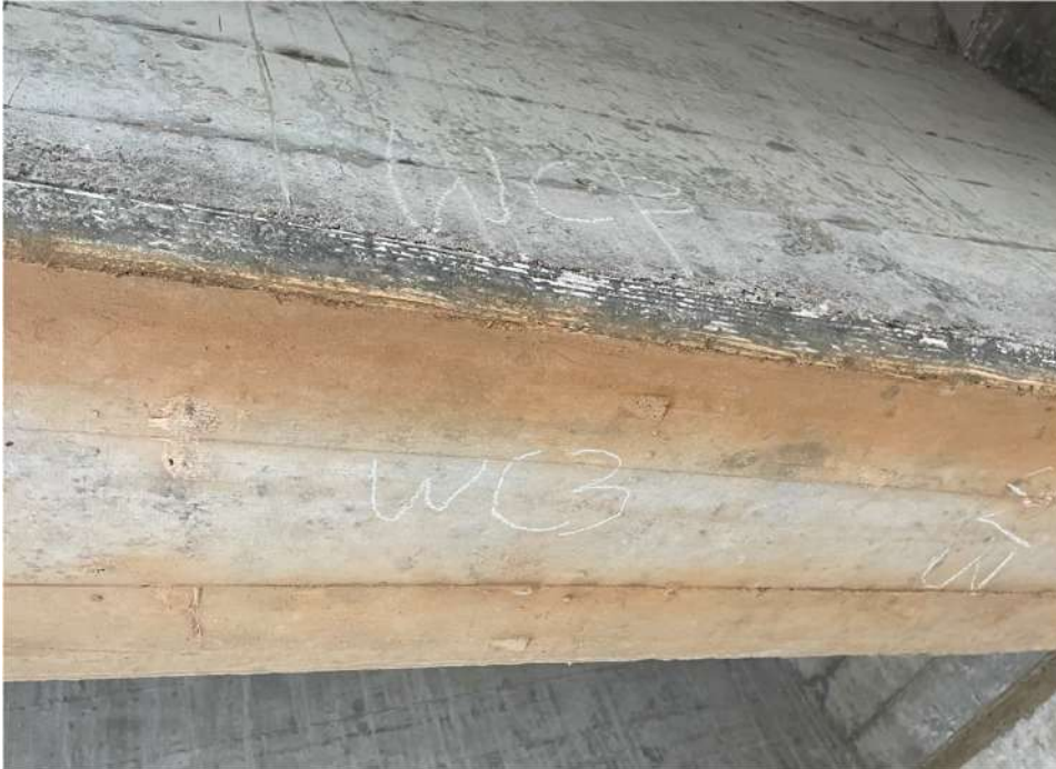
Photograph 11: Beam 3, cantilever span west, staining
