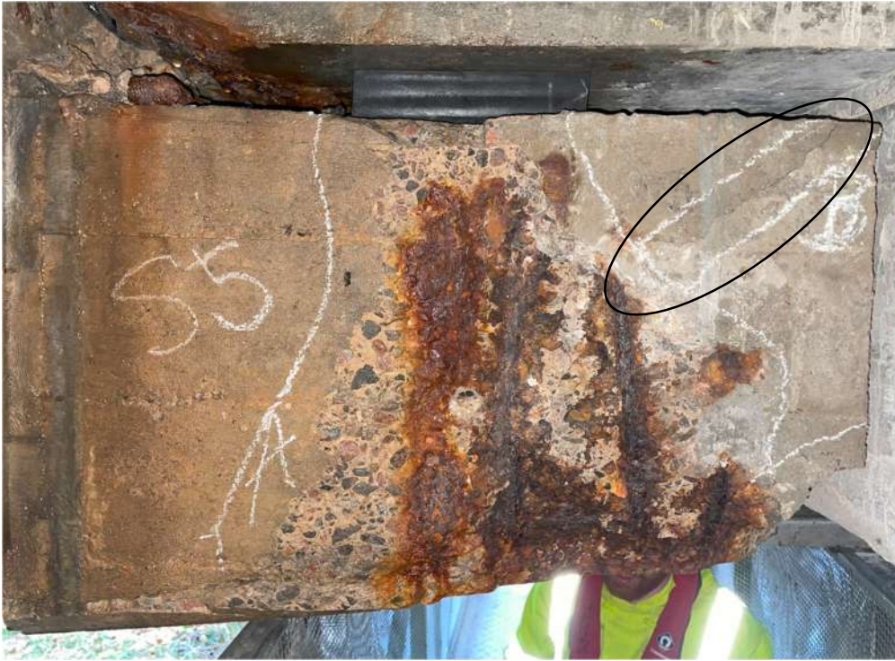
Photograph 73: Beam 5 (north facing), half joint east, crack running from spalled area to top corner
