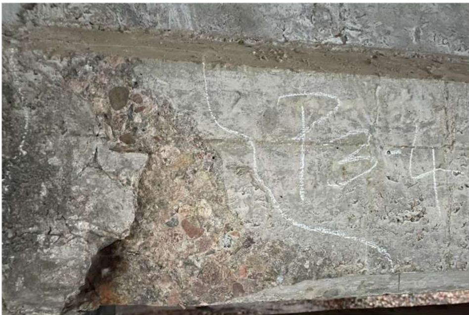
Photograph 78: Beam 3 – Beam 4, west pier, east face, spalled concrete with cracks extending from spall
