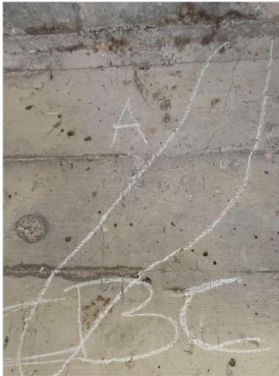
Photograph 76: Beam 2 – Beam 3 (both faces), central cross beam, hairline crack on diagonal from soffit of deck
