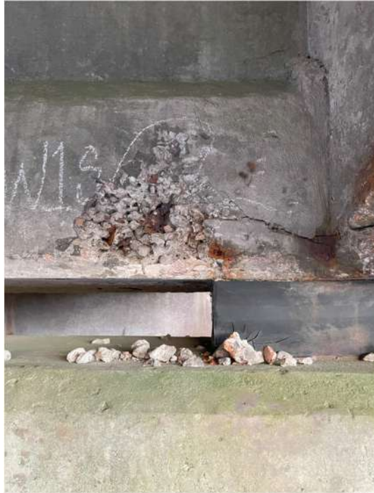
Photograph 77: Beam 1 – Beam 2, west pier, east face, spalling in area of large aggregate
