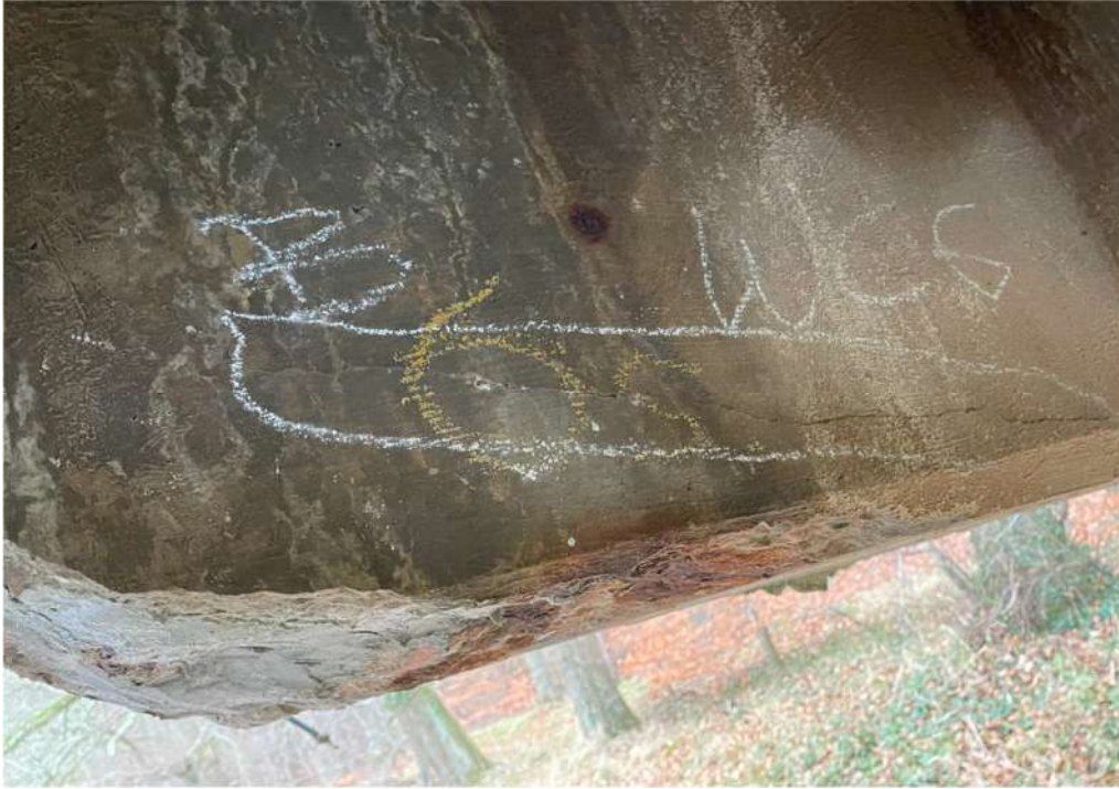
Photograph 55: Beam 6 (north facing), half joint west, crack, joins into Defect 54
