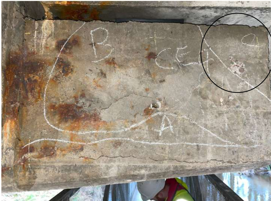
Photograph 68: Beam 4 (north facing), half joint east, cracking and spalling
