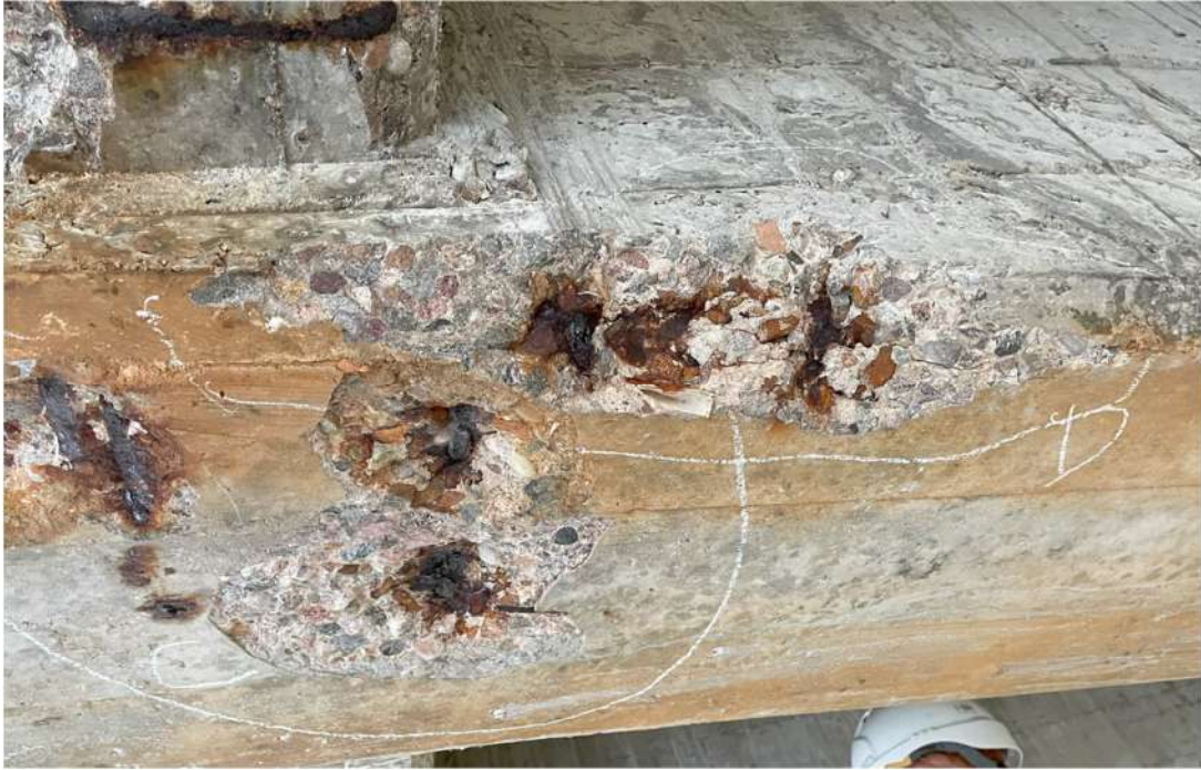
Photograph 13: Beam 3, cantilever span west, spalled concrete and reinforcement exposed
