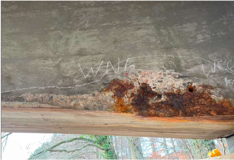
Photograph 15: Beam 6, cantilever span west, large spall
