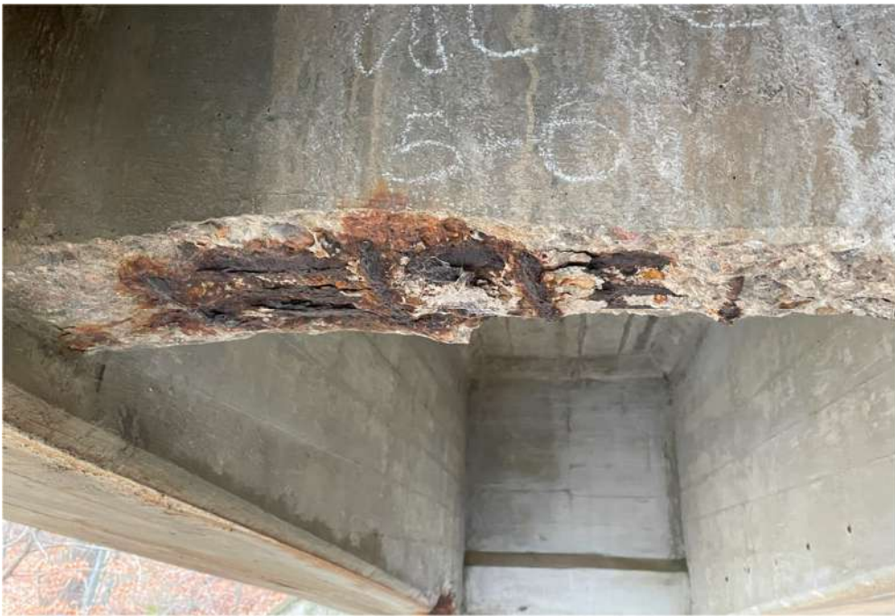
Photograph 20: Beam 5 – Beam 6, cantilever span west, cross beam, full width spall with exposed reinforcement
