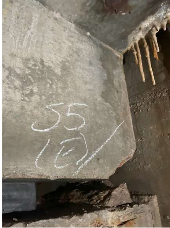
Photograph 69: Beam 5 (south and north facing), half joint east, spalling of corner, saturated and dripping
