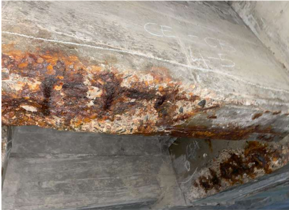
Photograph 33: Beam 4 – Beam 5, cantilever span east, crossbeam, full width spall with exposed reinforcement, full length crack through spall
