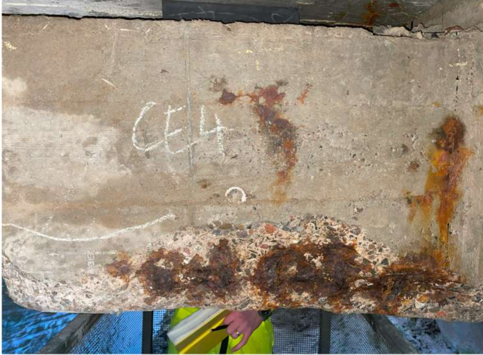
Photograph 65: Beam 4 (south facing), half joint east, spalling of bottom corner of beam, reinforcement exposed and corroded
