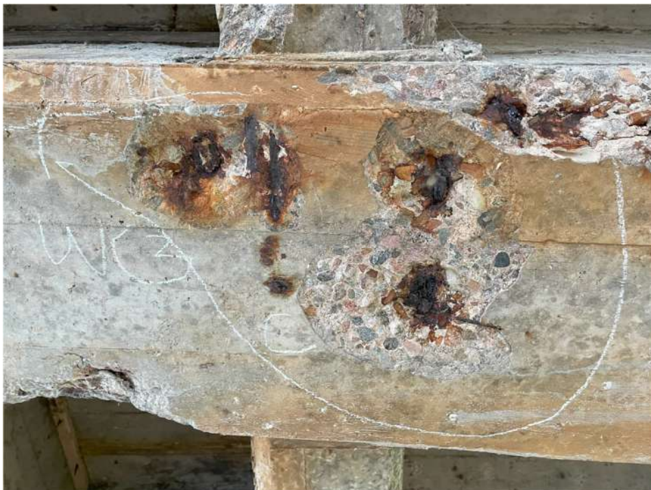
Photograph 12: Beam 3, cantilever span west, small spalls and reinforcement exposed
