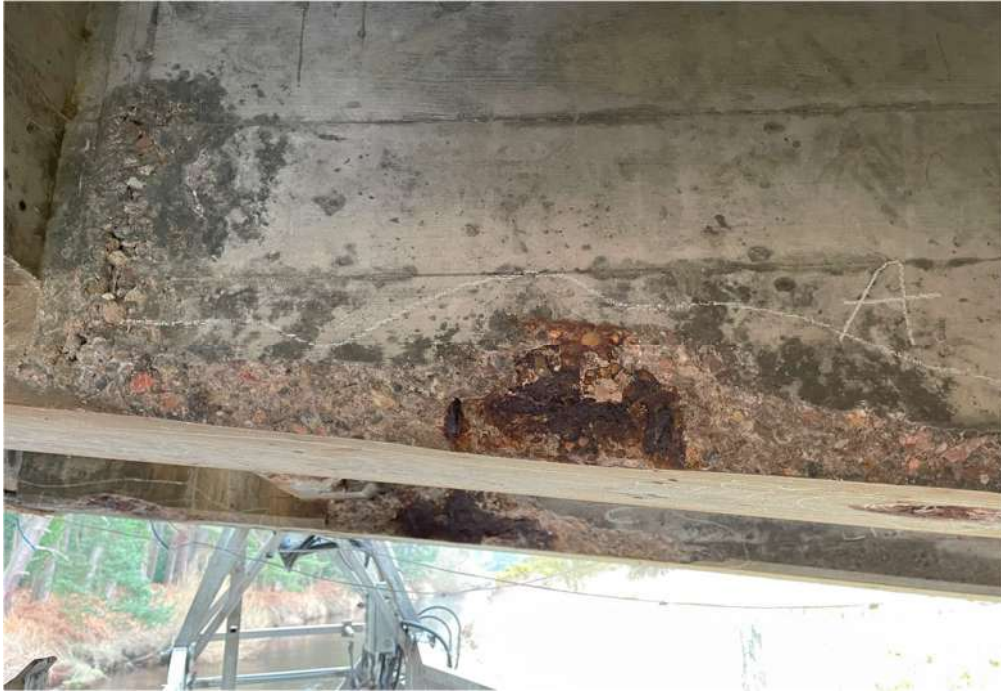
Photograph 25: Beam 2, cantilever span east, long spall, corner of beam is missing
