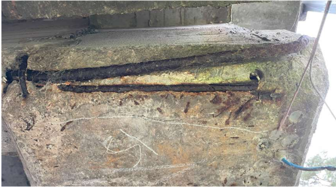
Photograph 59: Beam 1 (north and south facing), half joint east, end links exposed, one completely protruding and sheared
