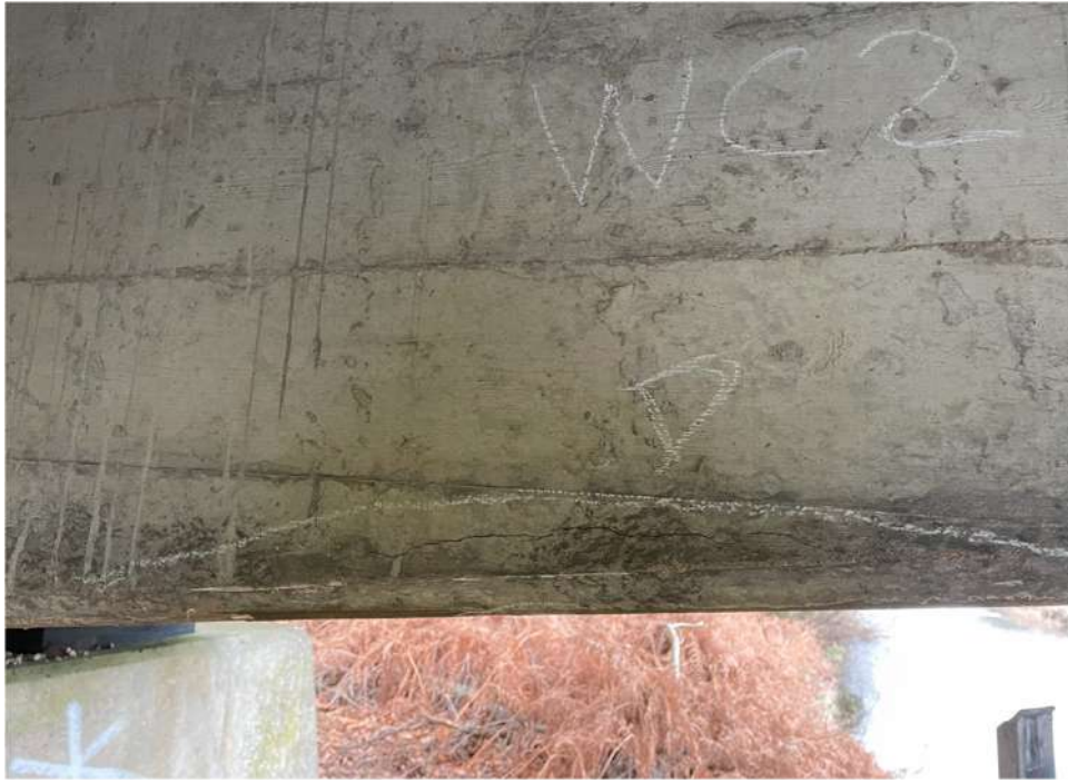
Photograph 7: Beam 2, cantilever span west, longitudinal crack
