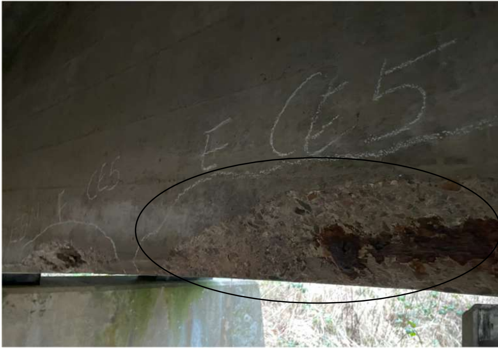
Photograph 27: Beam 5, cantilever span east, large spall reinforcement exposed and corroded
