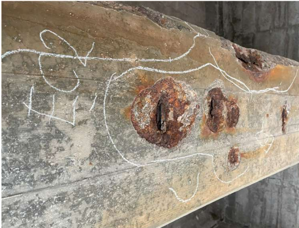
Photograph 24: Beam 2, cantilever span east, areas of small spalls and corrosion
