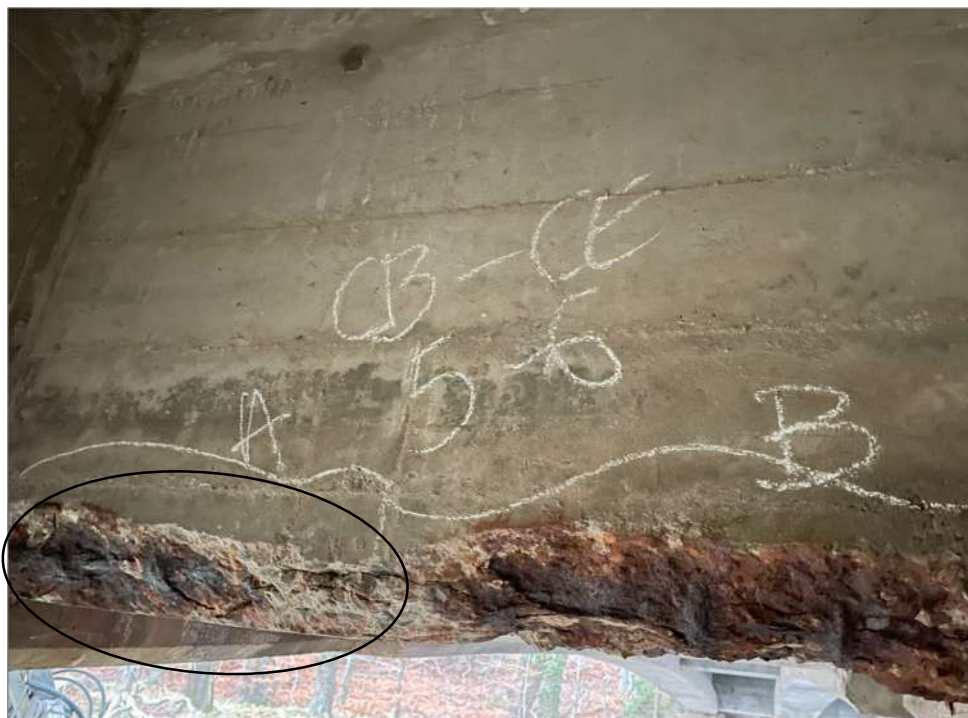
Photograph 34: Beam 5 – Beam 6, cantilever span east, crossbeam, spall with exposed reinforcement linked to defect 35
