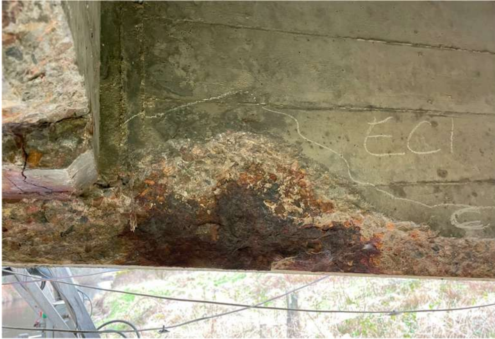
Photograph 23: Beam 1, cantilever span east. Large and deep spall, reinforcement exposed and corroded
