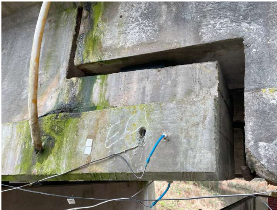
Photograph 58: Beam 1 (north facing), half joint east, water ingress with active water dripping and green mould on outside face
