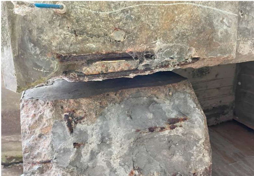
Photograph 56: Beam 6 (north facing), half joint west, spalling of soffit of end of suspended span, end links exposed
