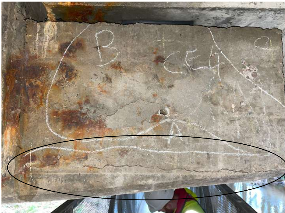
Photograph 66: Beam 4 (north facing), half joint east, spalling and cracking
