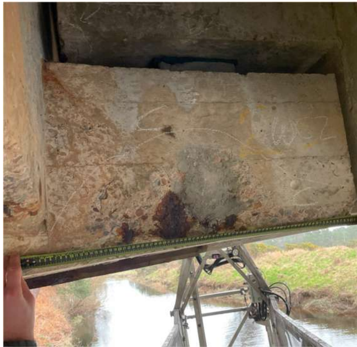
Photograph 44: Beam 2 (south facing), half joint west, loss of bottom corner section
