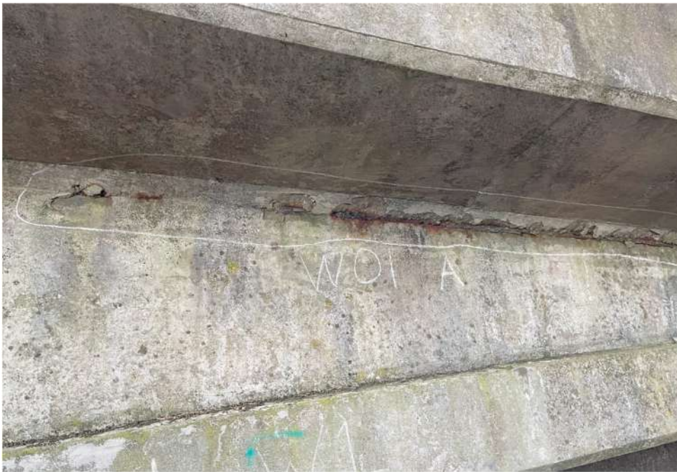
Photograph 37: Beam 1, outer span west, spalling along chamfer of the cantilever beam
