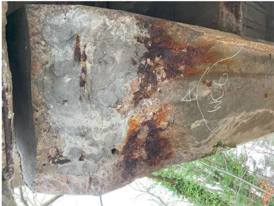
Photograph 54: Beam 6 (north and south facing), half joint west, large spall, previously repaired and corroded reinforcement exposed
