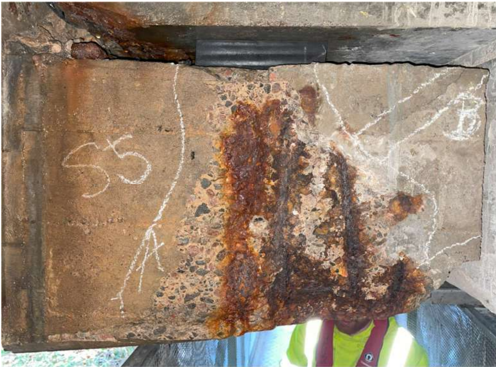
Photograph 72: Beam 5 (north facing), half joint east, significant spalling with exposed and corroded reinforcement
