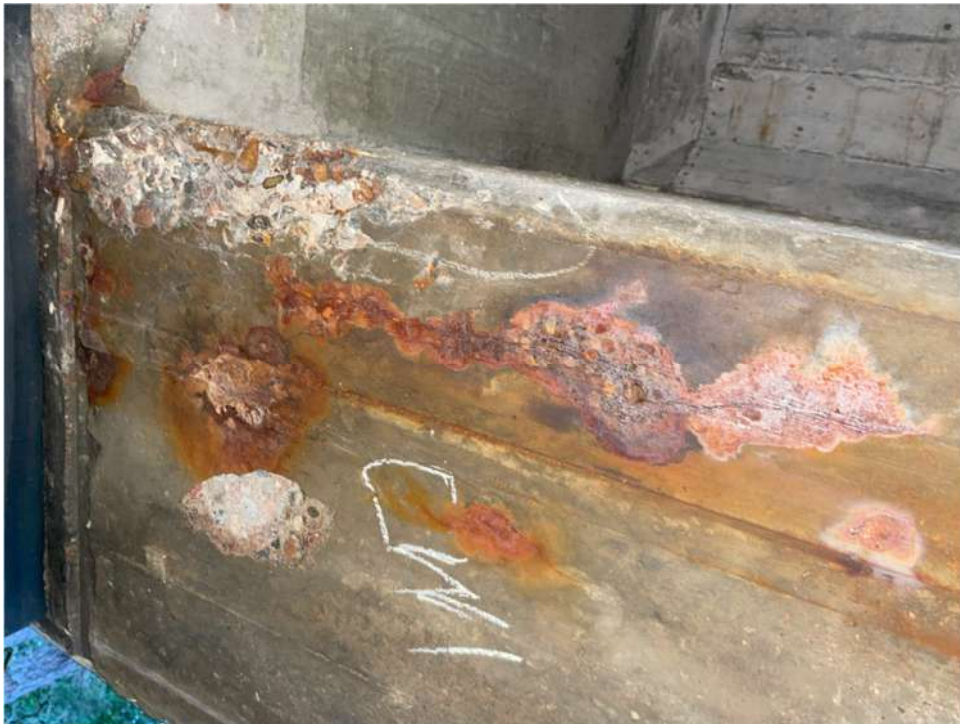
Photograph 4: Beam 1, cantilever span west, delamination and severe staining
