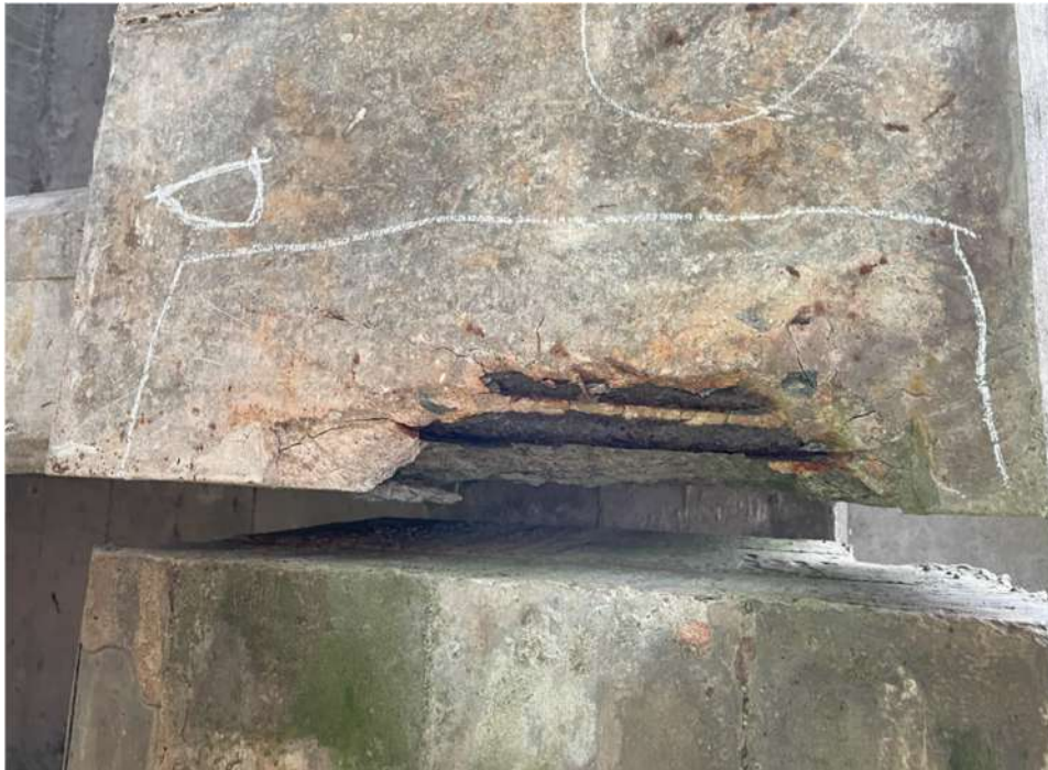
Photograph 40: Beam 1 (north and south facing), half joint west, severely corroded and exposed links, spall at end of beam
