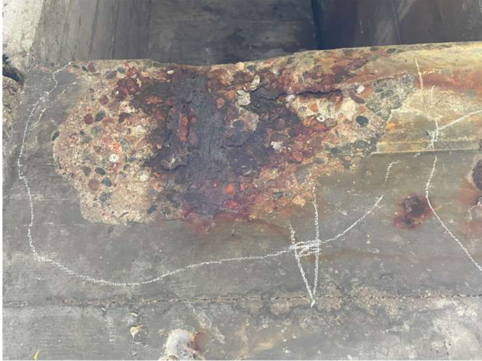
Photograph 21: Beam 1, cantilever span east, spalling on soffit of half joint
