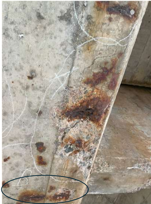
Photograph 6: Beam 2, cantilever span west, defect on bottom face of cantilever
