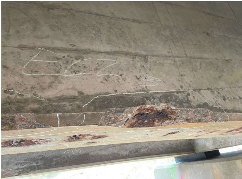
Photograph 26: Beam 2, cantilever span east, spalling concrete and staining
