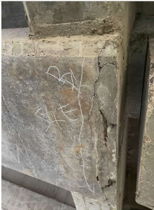
Photograph 64: Beam 4 (south facing), half joint east, spalling and cracking of soffit end of suspended span
