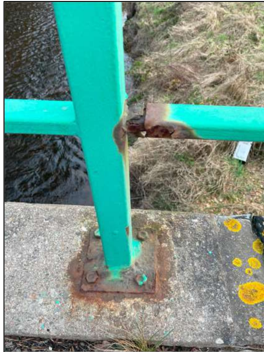
Fig 13. Localised paint failure at baseplates and guardrail join location
