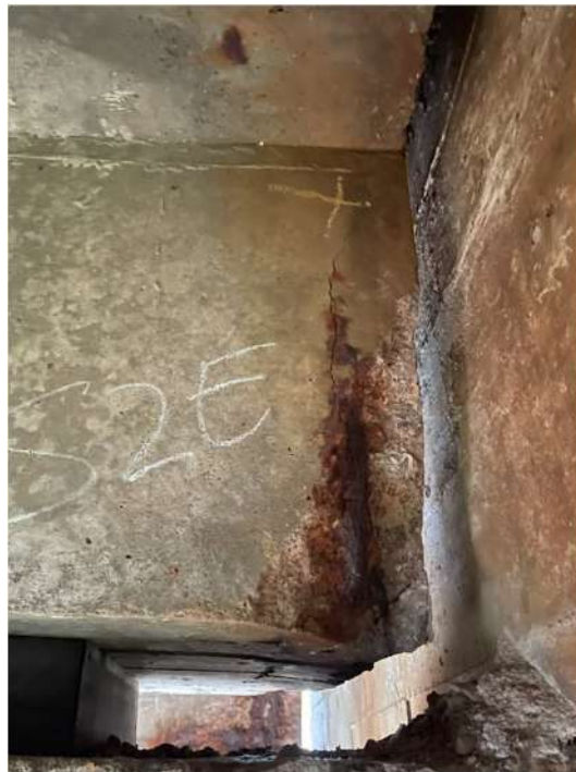
Photograph 60: Beam 2 (north and south facing), half joint east, end face link exposed, whole face is cracked with corner spalled
