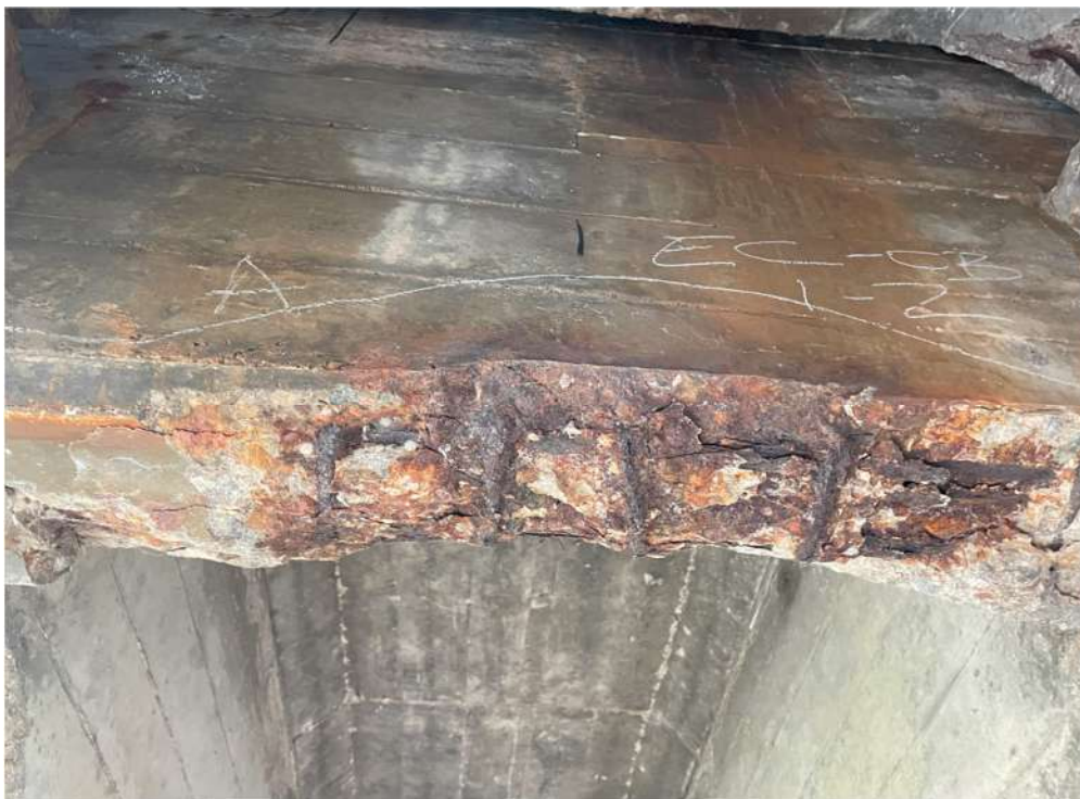
Photograph 32: Beam 1 – Beam 2, cantilever span east, crossbeam, full width spall with exposed reinforcement
