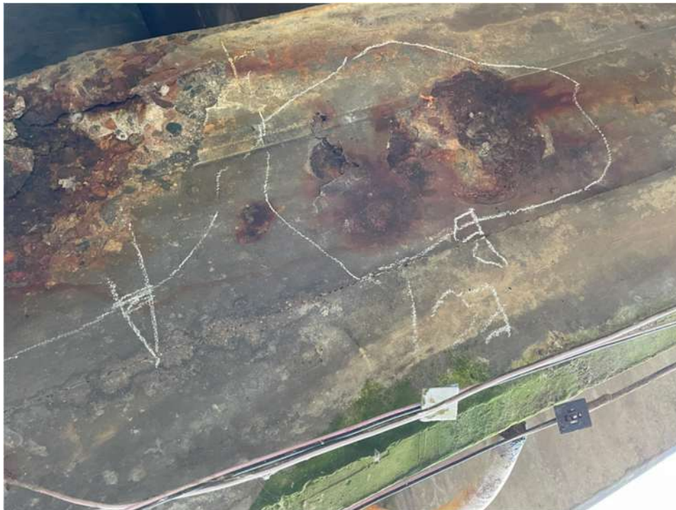
Photograph 22: Beam 1, cantilever span east, spalling and delaminating concrete
