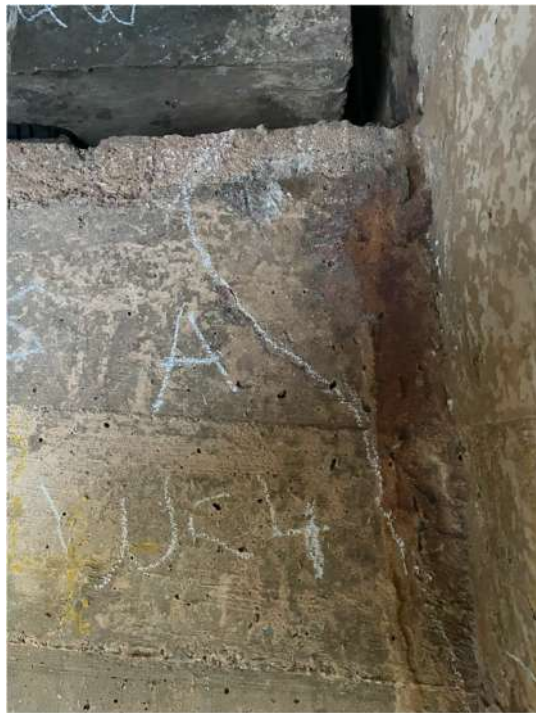
Photograph 48: Beam 4 (north facing), half joint west, hollow sounding and delamination
