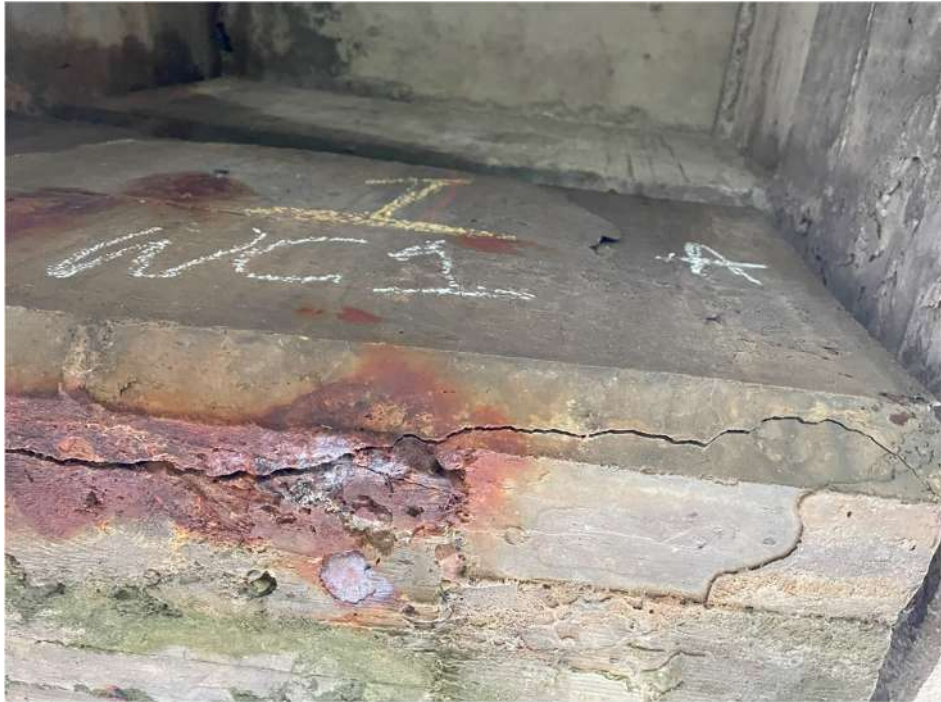
Photograph 42: Beam 1 (south facing), half joint west, delaminated face, beginning to spall, hollow sounding with large crack in bottom face
