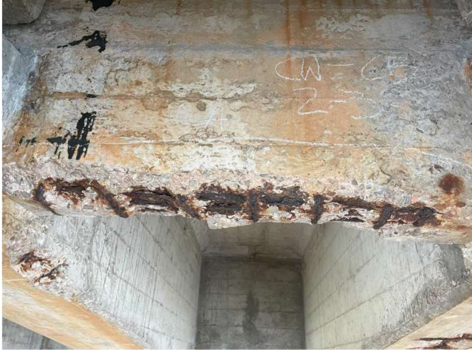
Photograph 17: Beam 2 – Beam 3, cantilever span west, cross beam, full width spall with exposed reinforcement
