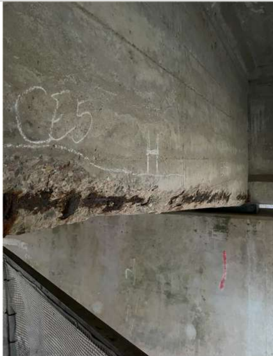
Photograph 30: Beam 5, cantilever span east, spall along bottom corner of beam, longitudinal reinforcement and links exposed
