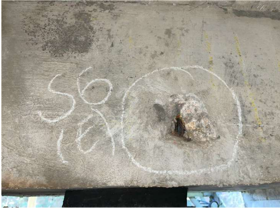
Photograph 75: Beam 6 (north facing), half joint east, isolated deep spall
