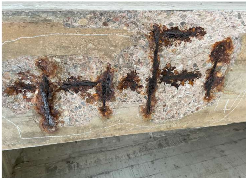
Photograph 8: Beam 2, cantilever span west, exposed and corroded reinforcement
