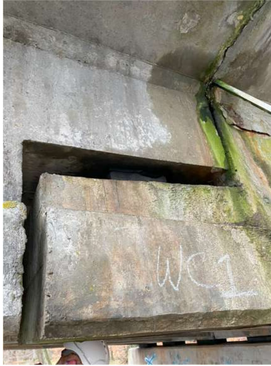
Photograph 41: Beam 1 (north facing), half joint west, Water ingress, damp and green mould on outside face
