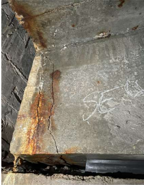
Photograph 63: Beam 4 (south and north facing), half joint east, end face corner cracker and spalling
