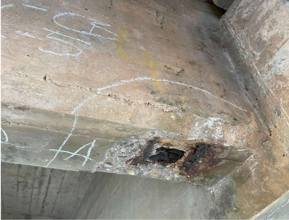
Photograph 19: Beam 4 – Beam 5, cantilever span west, cross beam, full width spall with exposed reinforcement
