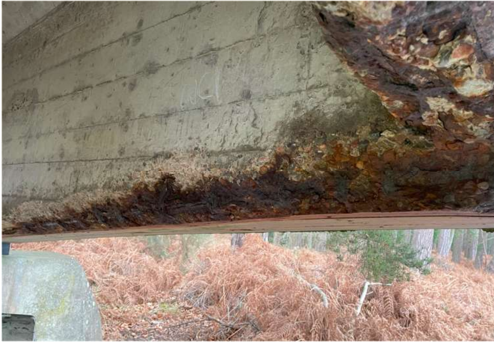
Photograph 3: Beam 1, cantilever span west, large spall
