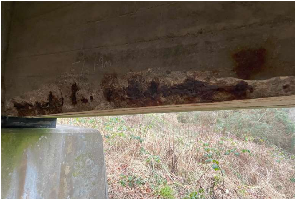
Photograph 31: Beam 6, cantilever span east, spall along bottom corner of beam, longitudinal reinforcement and links exposed
