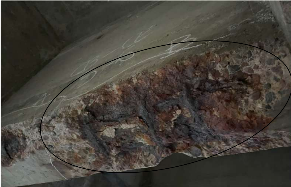
Photograph 35: Beam 5 – Beam 6, cantilever span east, crossbeam, full width spall with exposed reinforcement linked to defect 34
