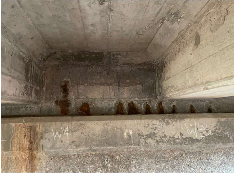
Photograph 83: Back face of abutment between beams, west abutment, delamination and general corrosion stains between beams, multiple spots
