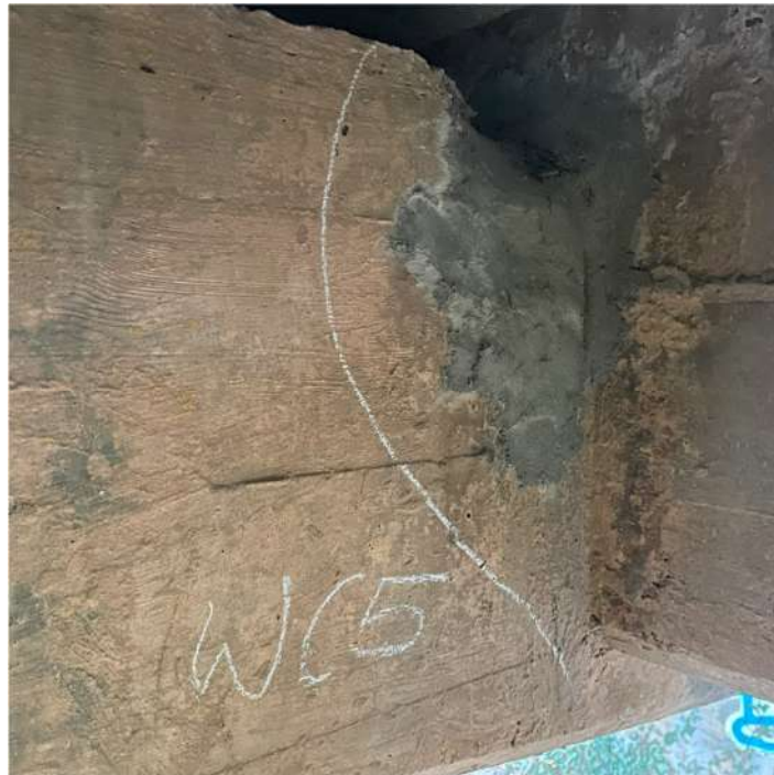
Photograph 52: Beam 5 (north facing), half joint west, area of missing concrete previous repair patch
