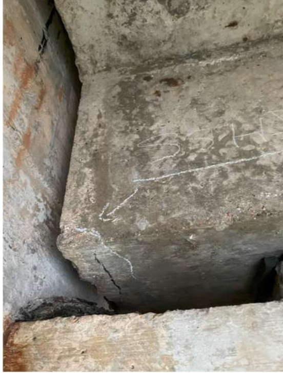
Photograph 43: Beam 2 (south facing), half joint west, crack and spalling
