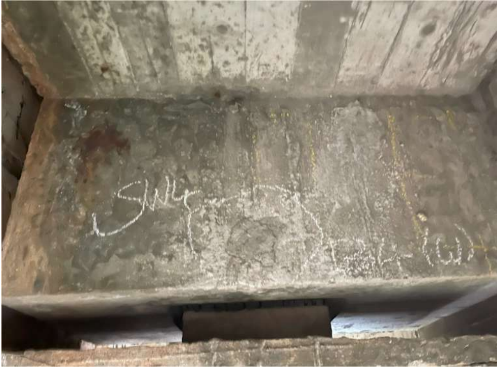
Photograph 49: Beam 4 (south facing), half joint west, patch repair
