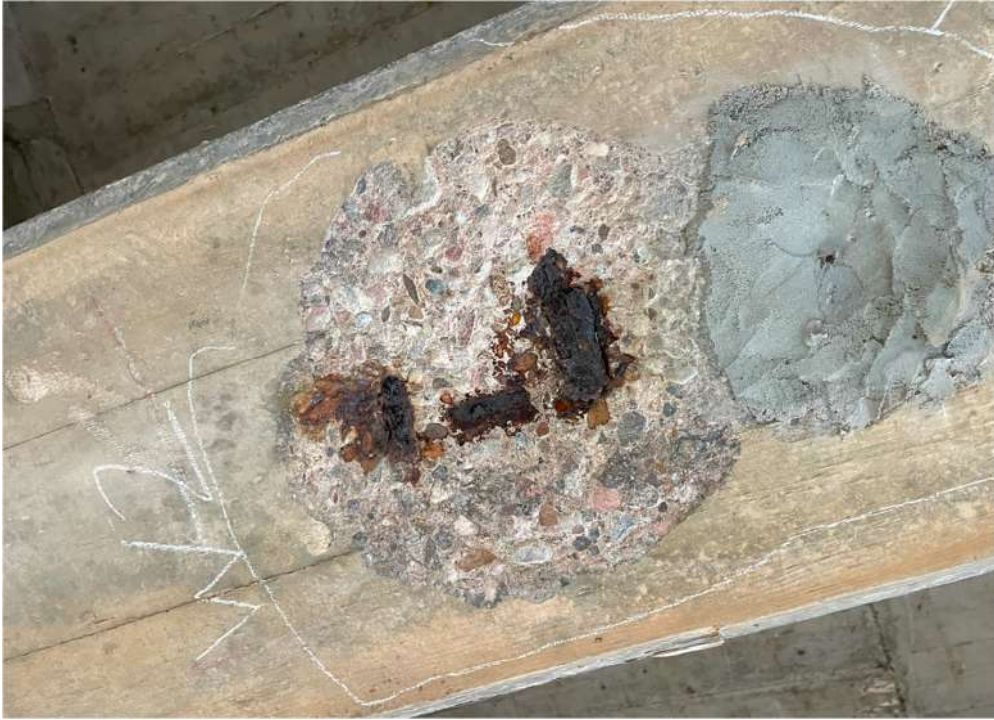
Photograph 9: Beam 2, cantilever span west, exposed and corroded reinforcement
