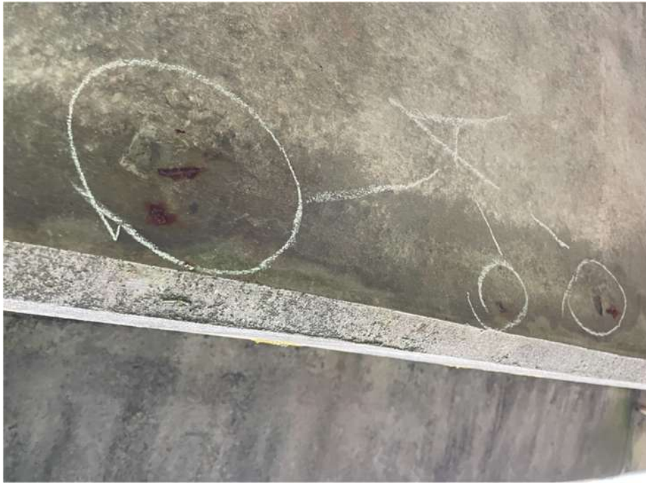
Photograph 1: Beam 1 soffit, suspended span, small corrosion spots
