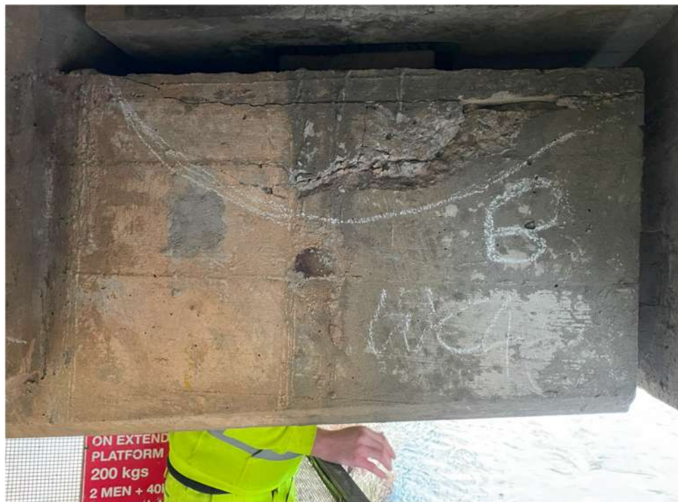
Photograph 50: Beam 4 (south facing), half joint west, crack below top face
