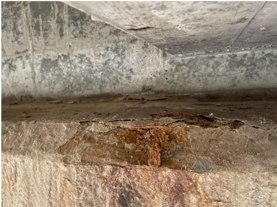
Photograph 82: Top of abutment, west abutment, delamination of top of abutment
