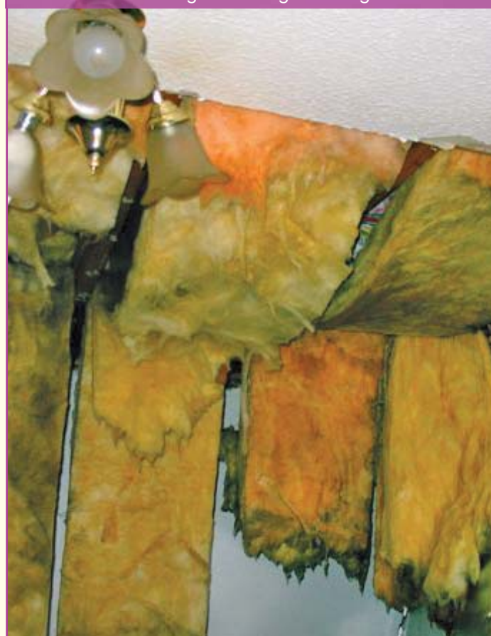
Water damage to ceiling following burst
