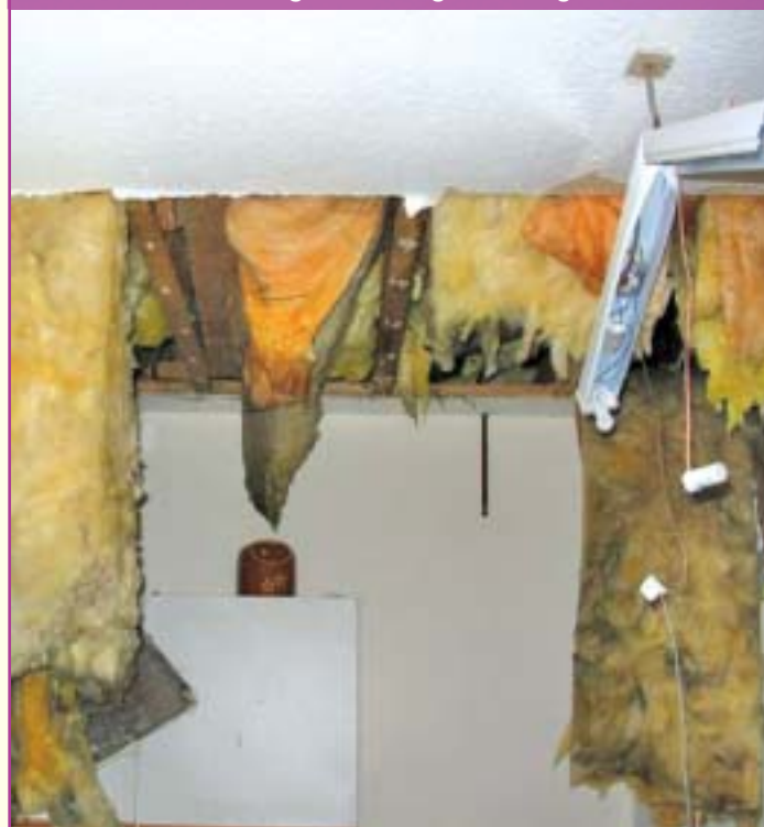
Water damage to ceiling following burst
