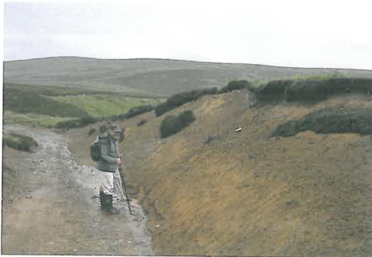
Plate 1: Stapler Road cutting in saprolite derived from deeply weathered and altered gabbro (Figure 13.6 of the ES)
