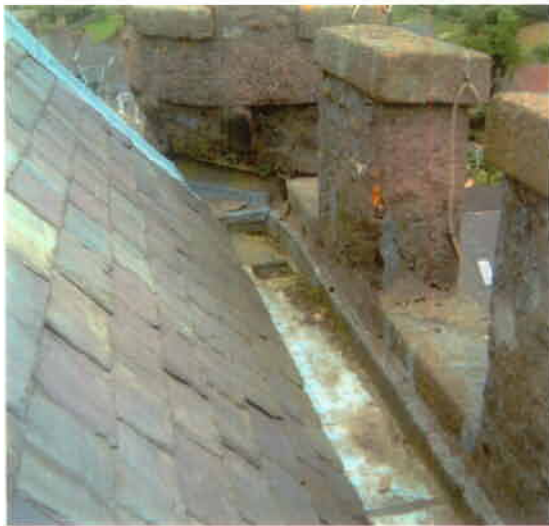
Photo 9 – South West Corner of Roof Gutter
