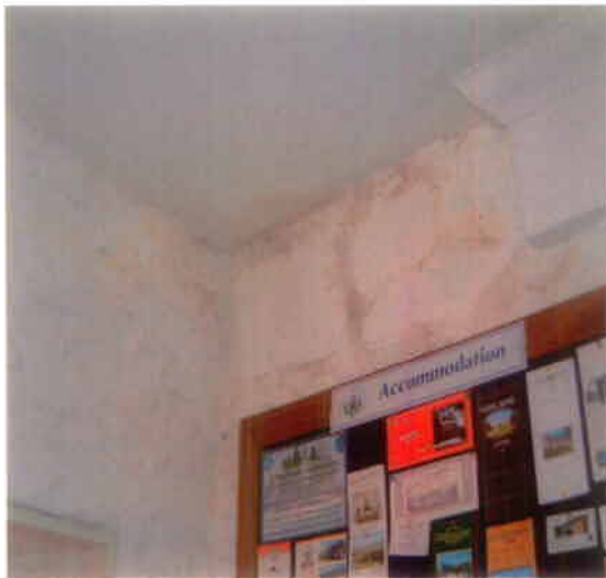
Photo 39 – Water Ingress NW Corner Ground Floor
