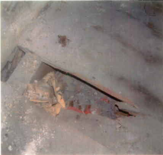
Photo 13 – Rotten Floorboard – Top Floor
