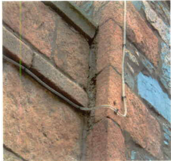
Photo 52 – Defective Pointing – NE Corner of Tower at Junction with Flat Roofed Section
