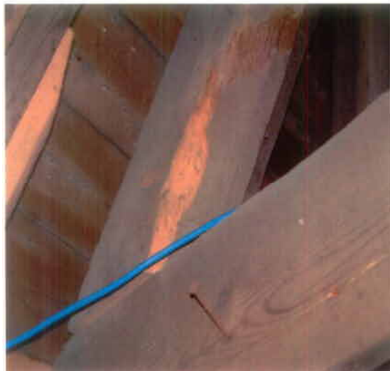
Photo 11 – Rotten Timber Rafter in Top Floor
