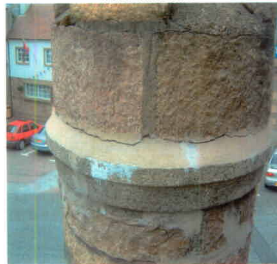
Photo 58 – Cracked Cement to Turret at NE Corner of Single Storey Roof
