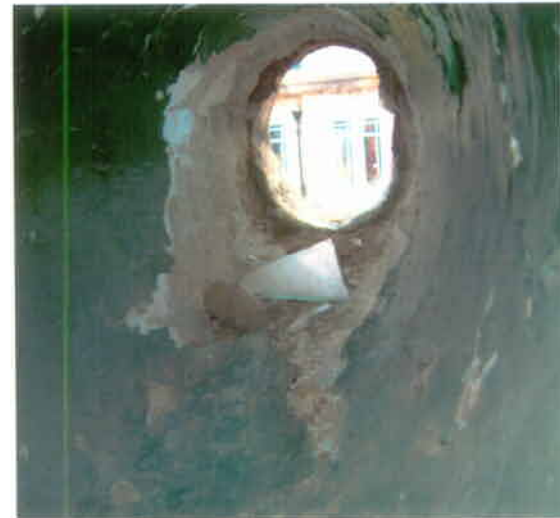
Photo 36 – Missing Glass to First Floor Staircase Peephole
