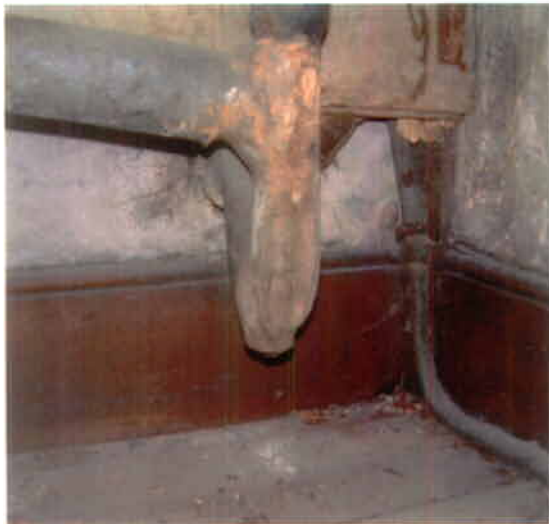
Photo 33 – Lead Pipework Below Sink
