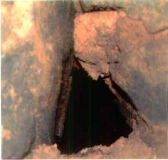
Photo 31 – Large Hole in West Wall
