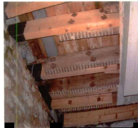
Photo 18 – Previous Joist Repairs to 3rd Floor Ceiling
