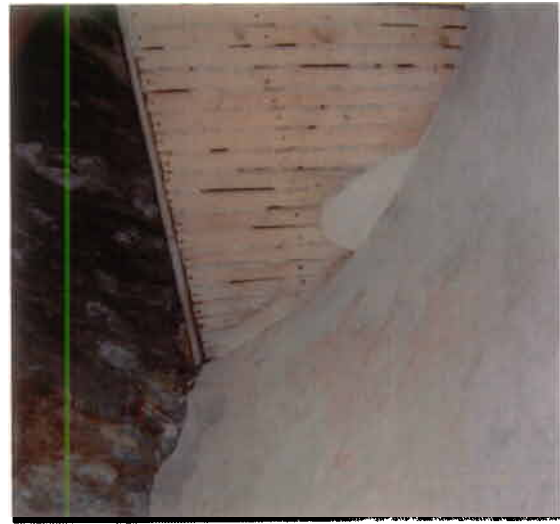
Photo 14 –Missing Plaster to Top Floor Stairwell
