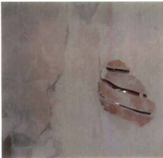
Photo 15 – Crack and Exposed Lath to Top Floor Stairwell
