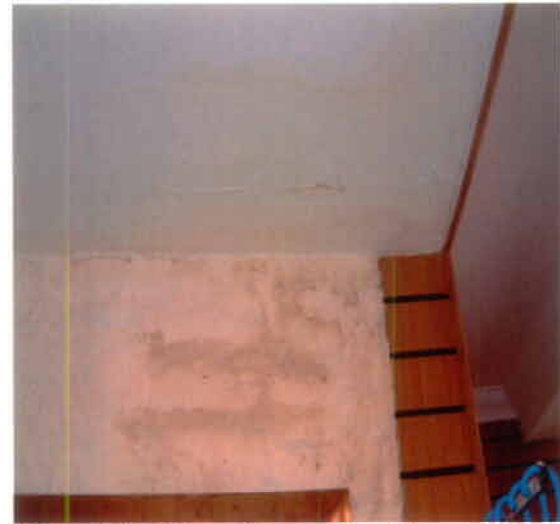
Photo 40 – Water Penetration Ground Floor Slapping
