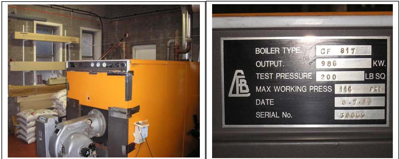
One of two existing oil boilers at Speyside High School
