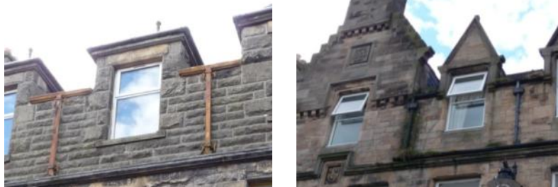
Damaged and poorly-maintained rainwater goods are common in the conservation area
