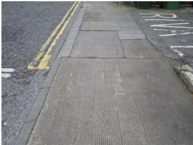
Poor quality surfaces in Mid Street
