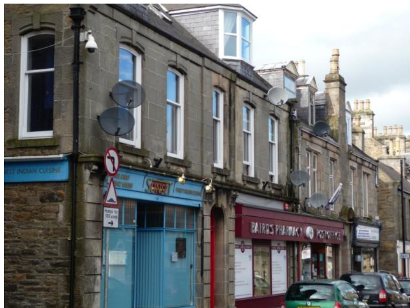
Small alterations such as satellite dishes can have a significant cumulative impact on character.
