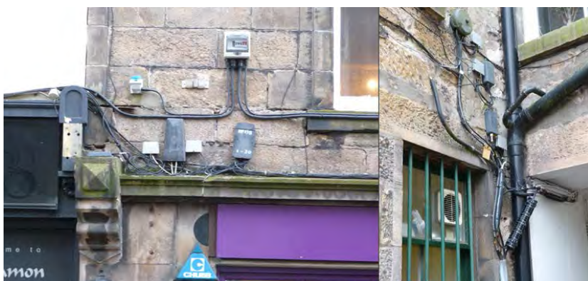
Untidy cables and cable boxes on buildings
