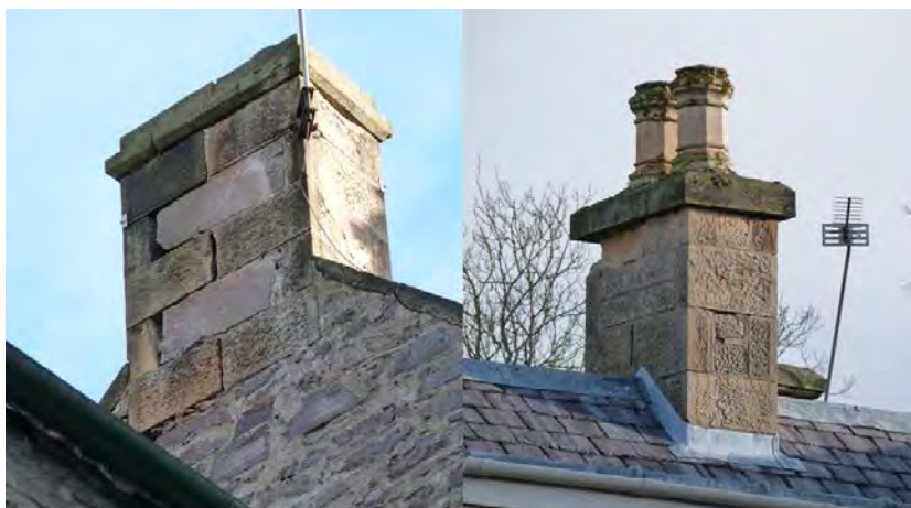
Instability in chimneyheads from missing pointing and stone decay
