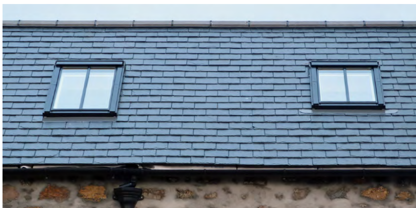
Roof reslated with new slates which are too black in colour and reflective; the ventilated ridge is a proprietary product for modern roofing systems and the 'conservation rooflights' are oversized and do not match the traditional rooflights found across the conservation area
