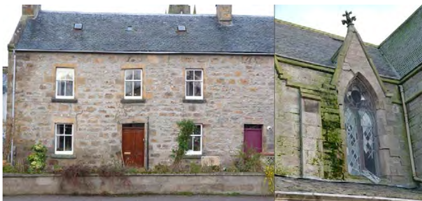
Façade showing distortion in lintols and cills from ground conditions and a gablet at the Castlehill Church showing structural distortion from the failure of an internal beam
