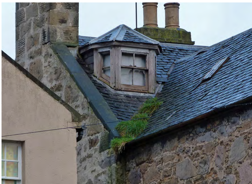
Valley gutter choked with vegetation causing dampness at the wallhead below, slipped slates and woodwork not maintained or decorated
