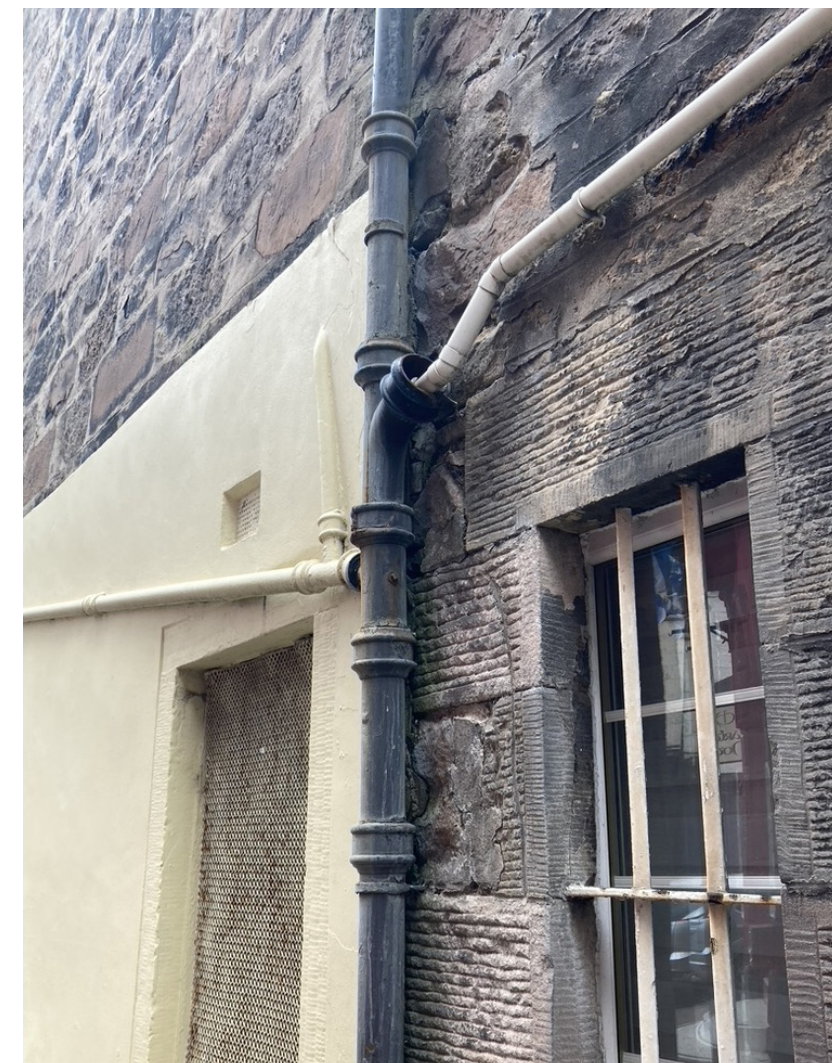
This detail shows a mixture of cast iron and uPVC with miss-matched sizing - drainage rather than rainwater, but not ideal.
