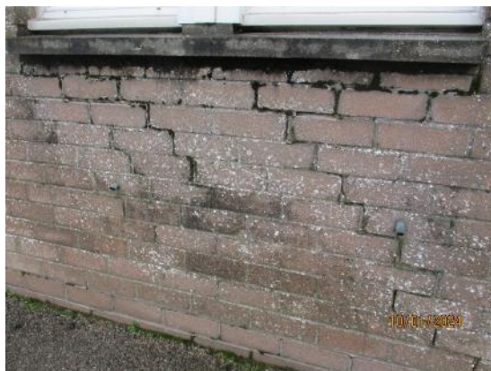
24. Cracking to brickwork walls
