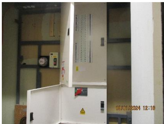
165. Main swiychboard – distribution 1/6 Cupoard
