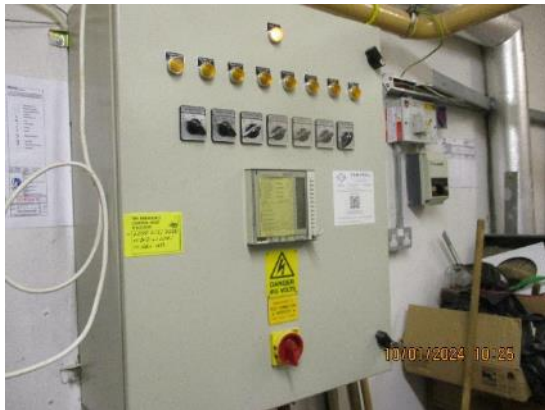
173. Control panel – heating system. Boiler house.
