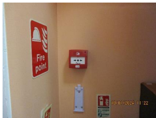
184. Fire alarm call point. Typical.
