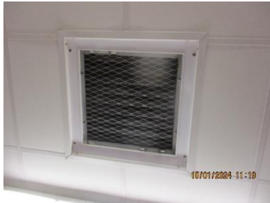
164. Kitchen extract internal grille.
