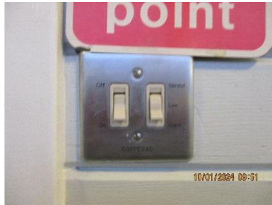
174. Convactor heater – switch control typical.
