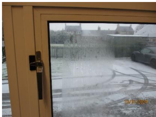
48. Fogged double glazed units
