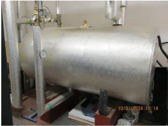
155. Hot water storage calorifier boiler house.
