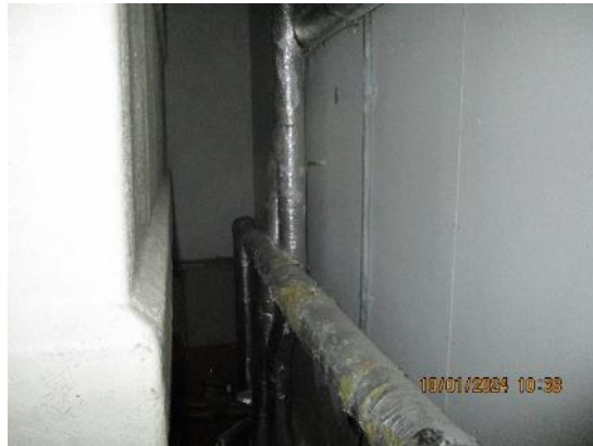
158. Cold water pipework in tank room.
