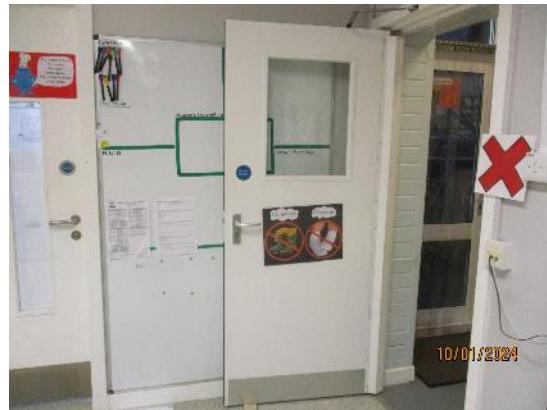
109. Timber solid core fire doors
