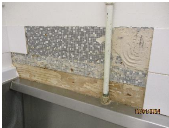
101. Missing ceramic tiles – Boys toilet
