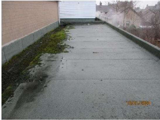
19. Blocked box gutters
