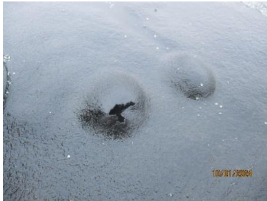
9. Punctured blisters in bitumen repairs
