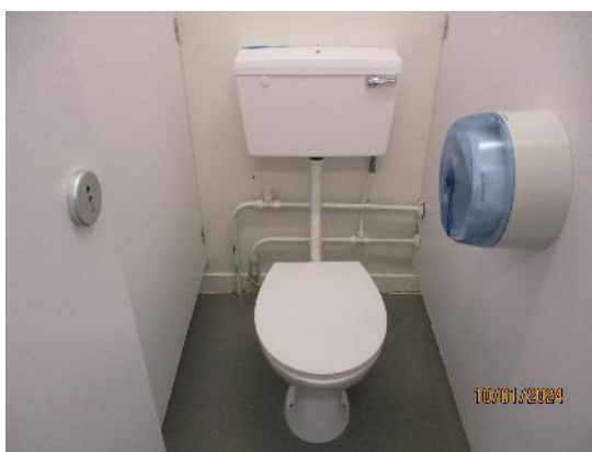
117. Pupil toilets with PVC cisterns
