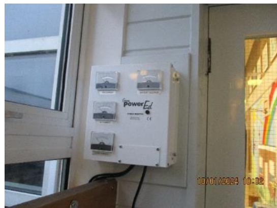
172. Solar panel voltage monitoring unit. 1/16 corridor
