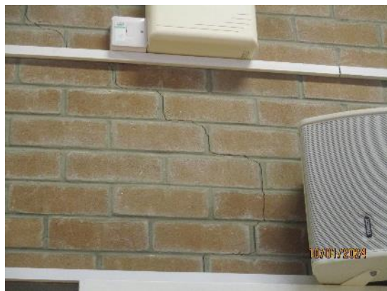
89. Cracking to Games Hall
