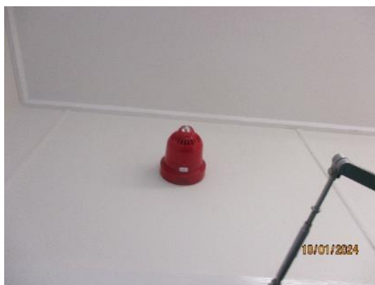
186. Fire alarm sounder beacon boys toilet 1/11 typical.
