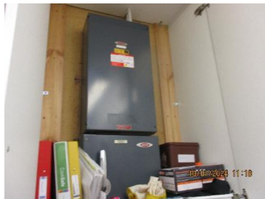
166. DB and isolator – kitchen cupboard.
