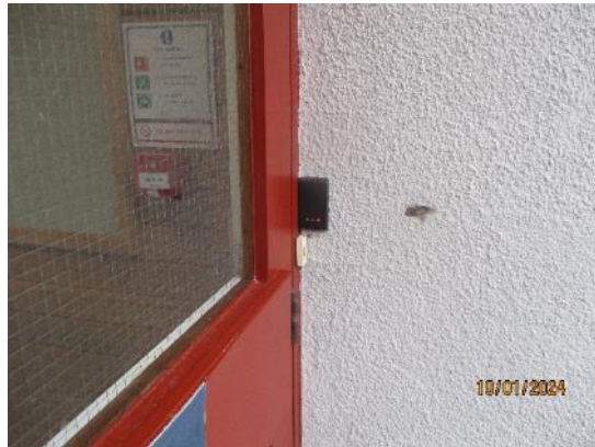
194. Door entry card reader. 1/12 external door.
