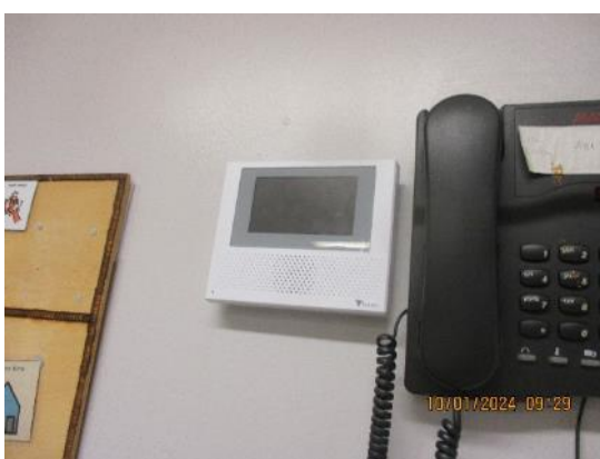
190. Door entry system monitor nursery class 1/15.
