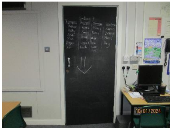
105. Timber hollow core store doors
