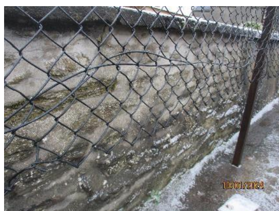
213. Damage to chain link fencing
