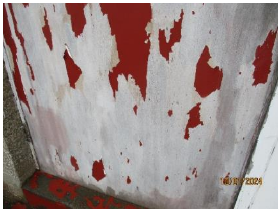
57. Timber external doors peeling
