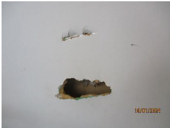
108. Isolated damage to hollow core doors
