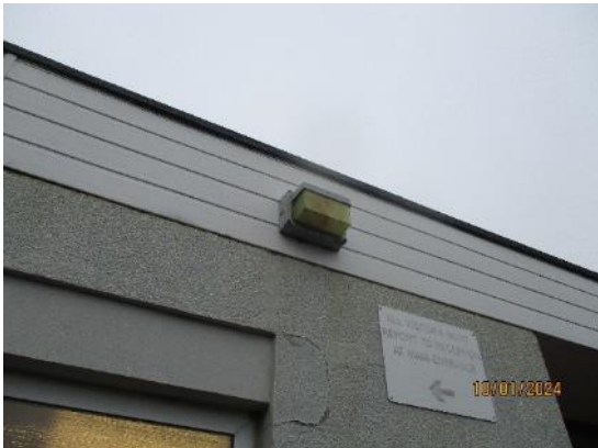
181. External lighting typical.
