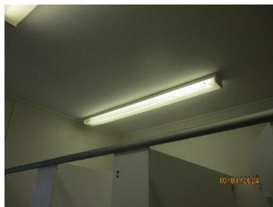
178. Lighting – girls toilet 1/10
