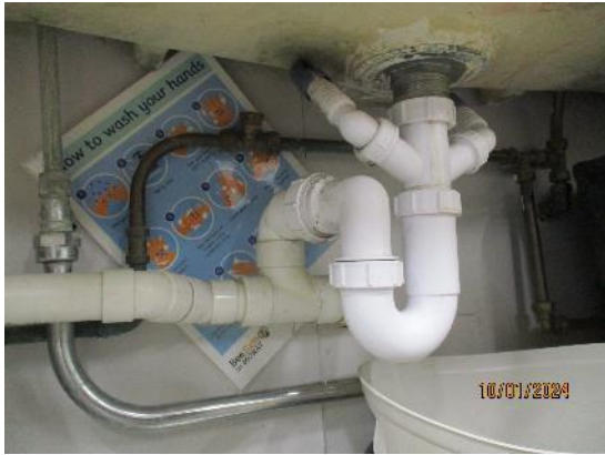
137. PVC waste pipes
