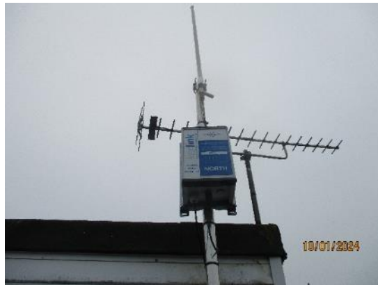
192. Internet receiver unit – roof mounted.
