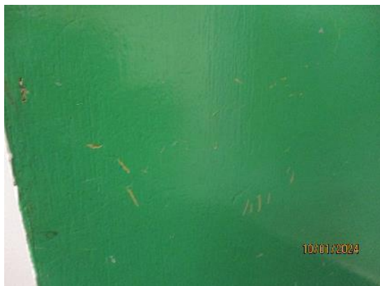
140. Scratched timber doors
