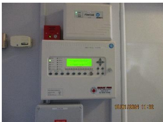
185. Fire alarm control panel and radio hub 1/1 corridor
