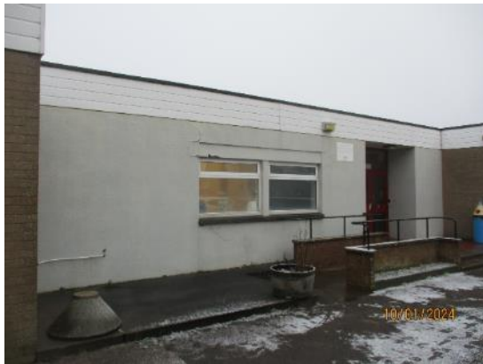
55. Flaking paint on rendered wall
