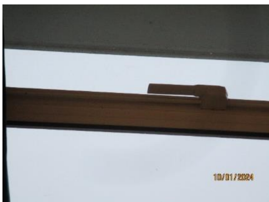
53. High level latches operated by winding handles
