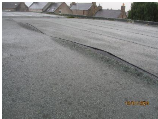
6. Raised seams in felt roofing
