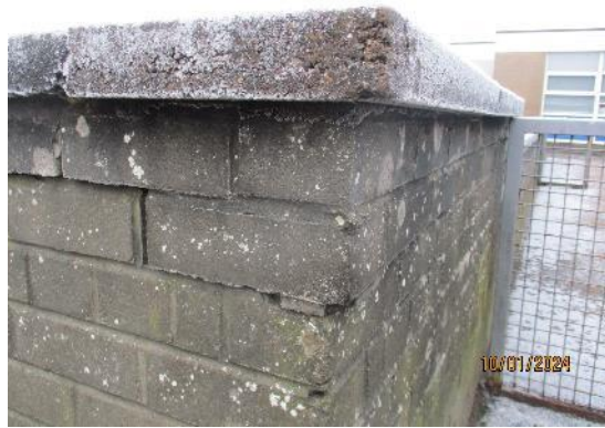
222. Impact damage to brick walls
