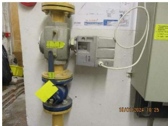
160. Gas supply main solenoid valve. Boiler house.
