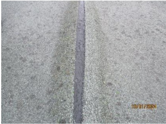
7. Open seams in felt roofing
