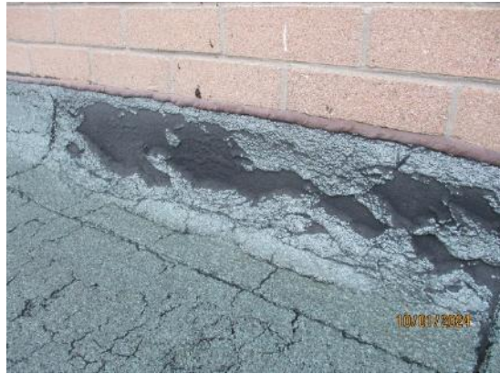
8. Surface erosion of felt flashings
