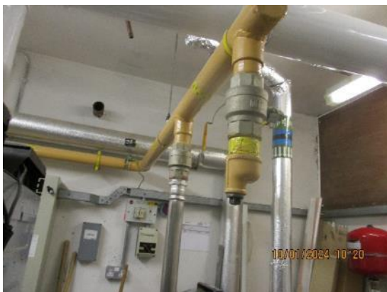
159. Gas supply pipework at boilers.
