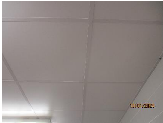
85. Suspended ceiling tiles - Kitchen
