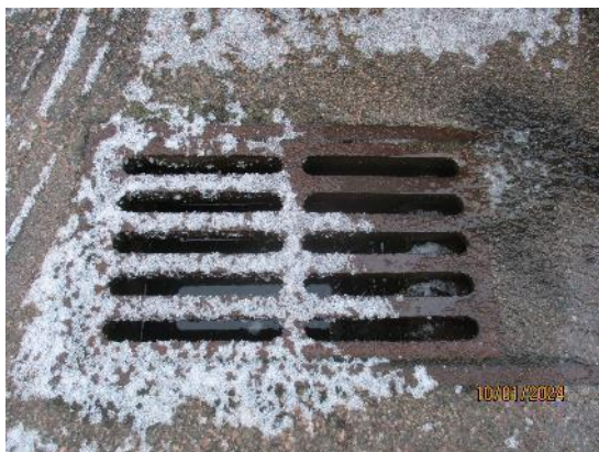
232. Car park road gully drainage
