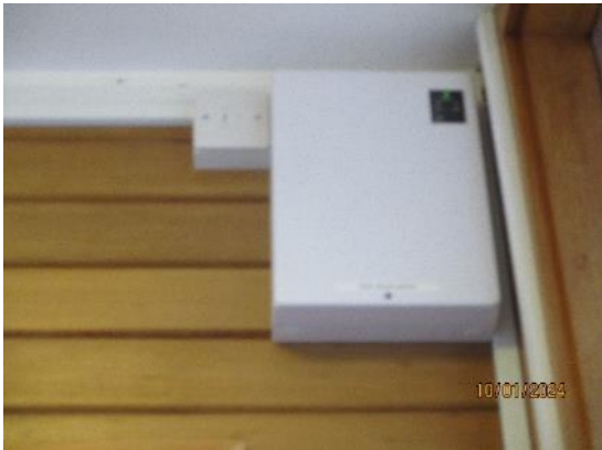
193. Door entry system control panel. 1/12 lobby.
