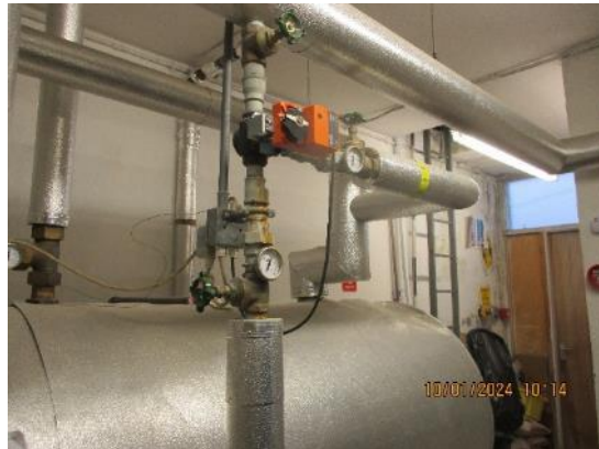
152. Heating primary pipework – boiler house.
