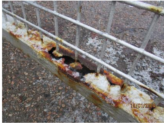
216. Metal frame corrosion
