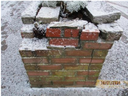
223. Impact damage to brick walls
