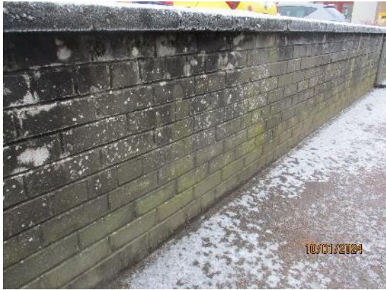
221. Impact damage to brick walls
