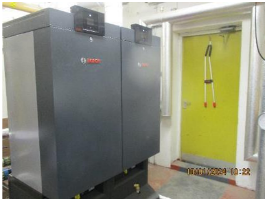
149. Natural gas high efficiency boilers
