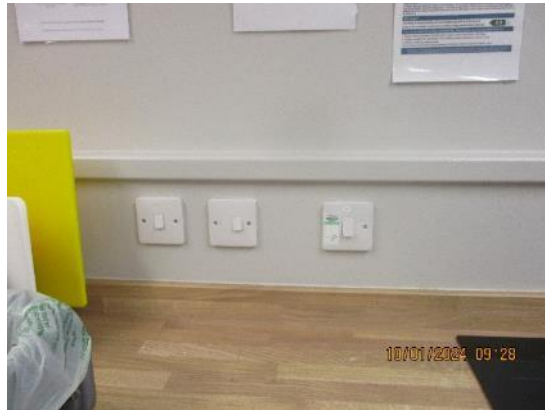
170. Switches – new nursery typical.
