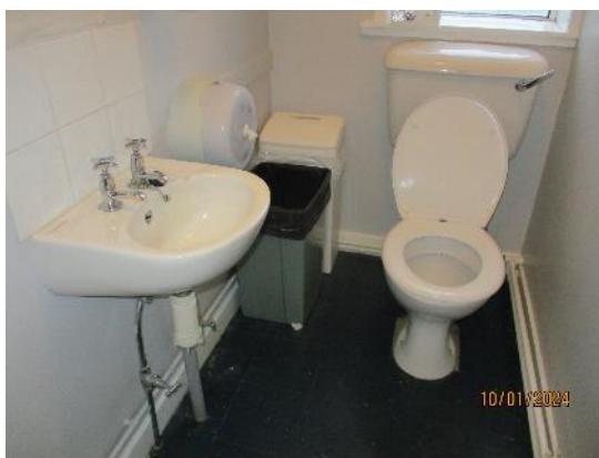
119. Staff toilets with china cisterns
