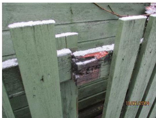
210. Damaged timber fencing
