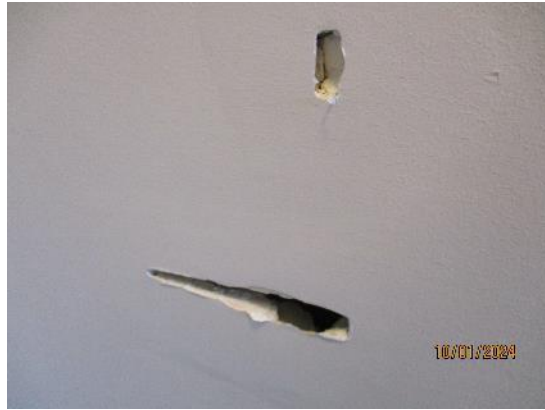
97. Door handle damage to plasterboard
