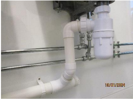
126. PVC waste pipes
