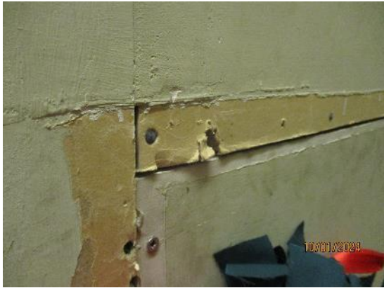
96. Isolated damage in Store Rooms
