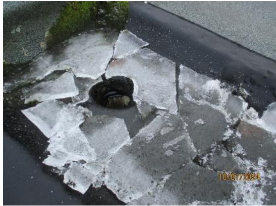
20. Missing balloon gratings
