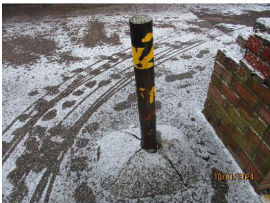
201. Loose steel bollard
