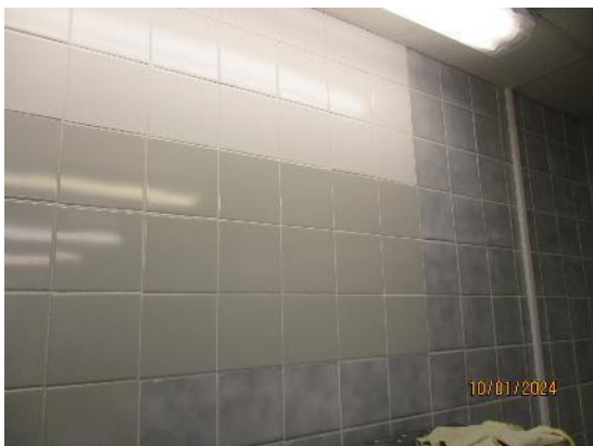
100. Ceramic tiles with patch repairs
