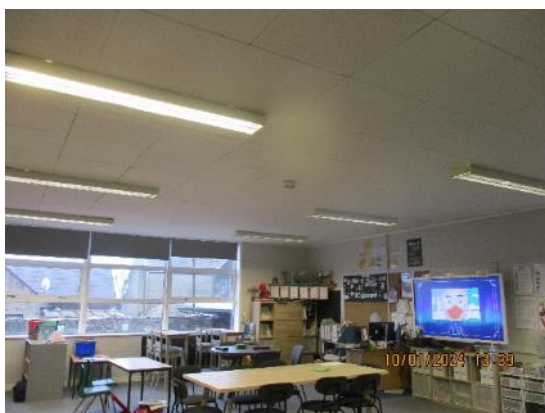
177. Lighting – classroom typical. 1/13
