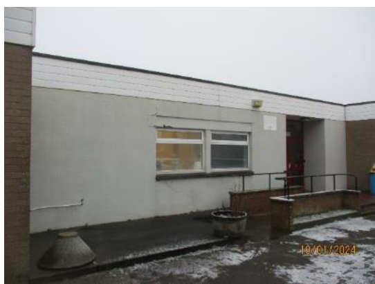
34. Cracked render finish
