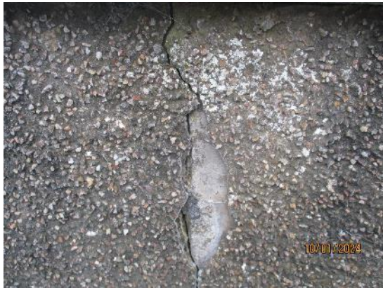
230. Roughcast cracking and spalling
