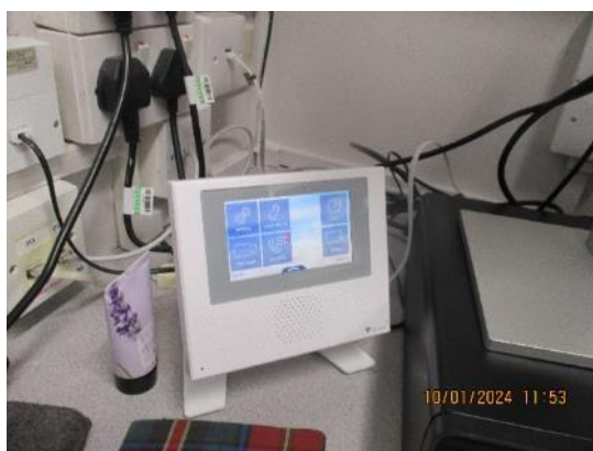
188. Door entry system monitor and handset – reception office 1/7 for main entrance.
