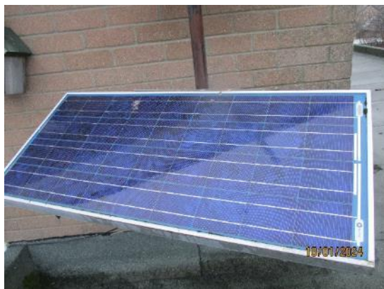
171. Solar PV panel – roof mounted.
