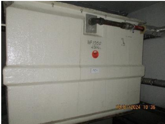
157. Cold water storage tank – above boiler house.
