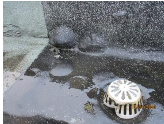
16. Blistered previous repairs
