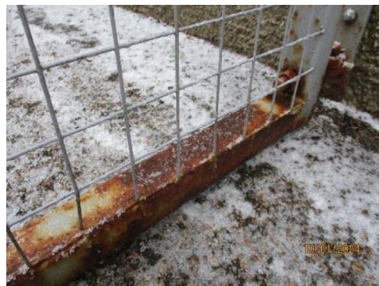
60. Surface corrosion to steel gates
