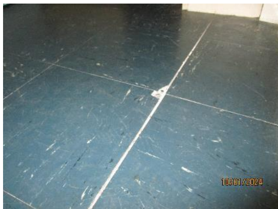
77. Chipped and broken vinyl tiles
