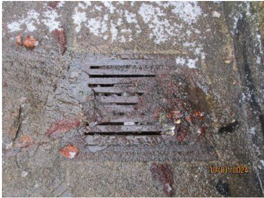
233. Playground drainage partially blocked
