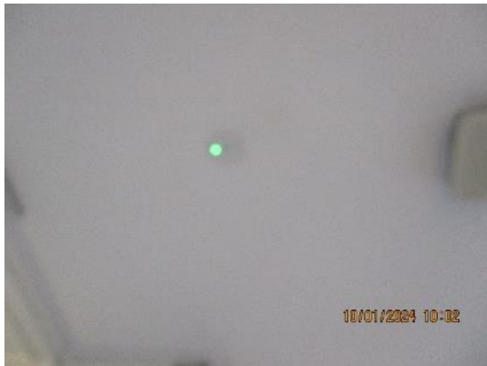
179. Emergency LED lighting. Nursery corridor 1/16
