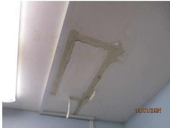
87. Water damaged plasterboard ceiling
