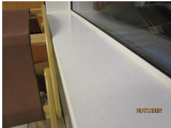
103. Timber window sills blistered and water marked
