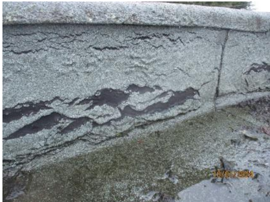
10. Cracking and surface erosion of upstands
