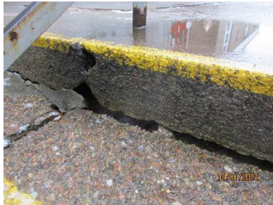
206. Gaps in concrete steps
