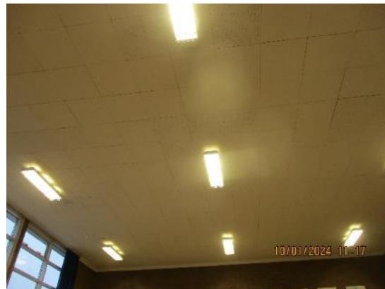
176. Lighting – main hall. 1/21
