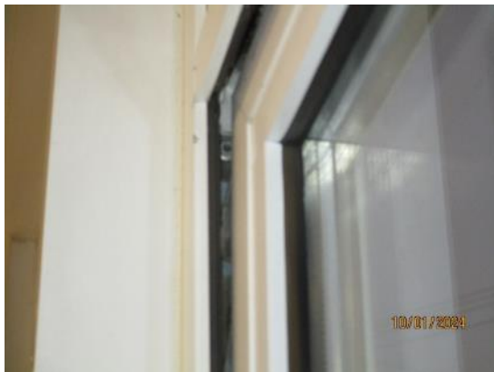
52. Faulty mechanism not sealing when closed
