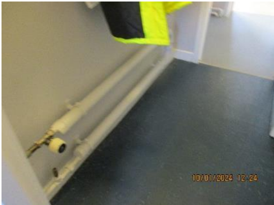
151. Heating system pipework in staff toilet.
