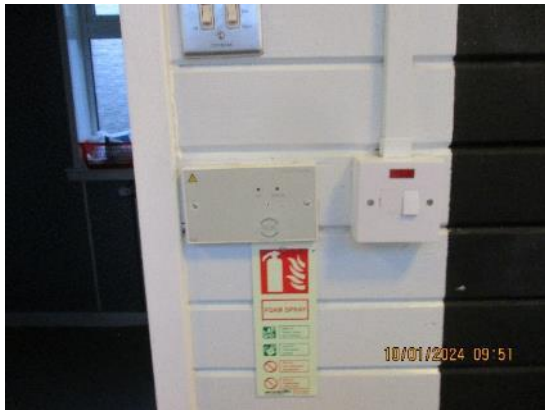
191. Disabled toilet alarm system panel WC 1/19
