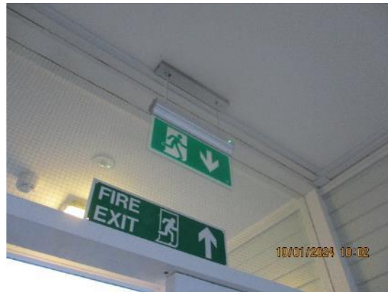
180. Emergency exit sign light 1/16 to 1/20 lobby.
