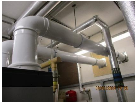
150. Boiler individual flue pipes
