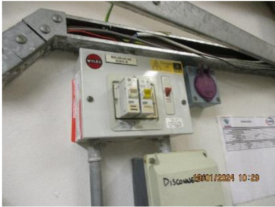
167. DB – 2 way 1 phase – boiler house.
