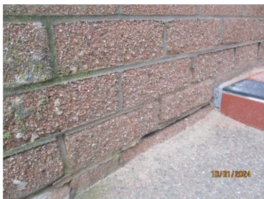
32. Isolated surface erosion
