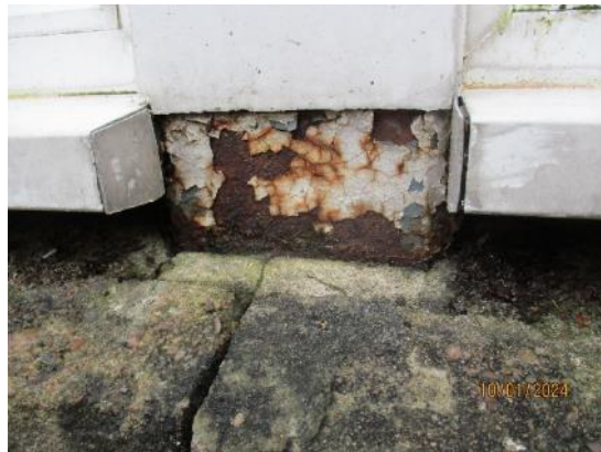
56. Surface corrosion to Courtyard steel frame
