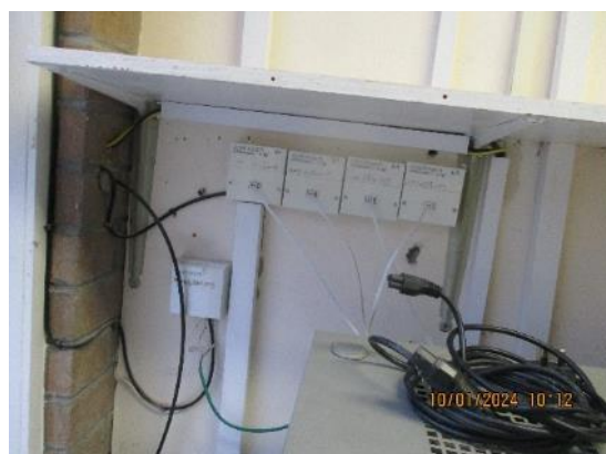
187. BT incoming phone line and distribution boxes. 1/23
