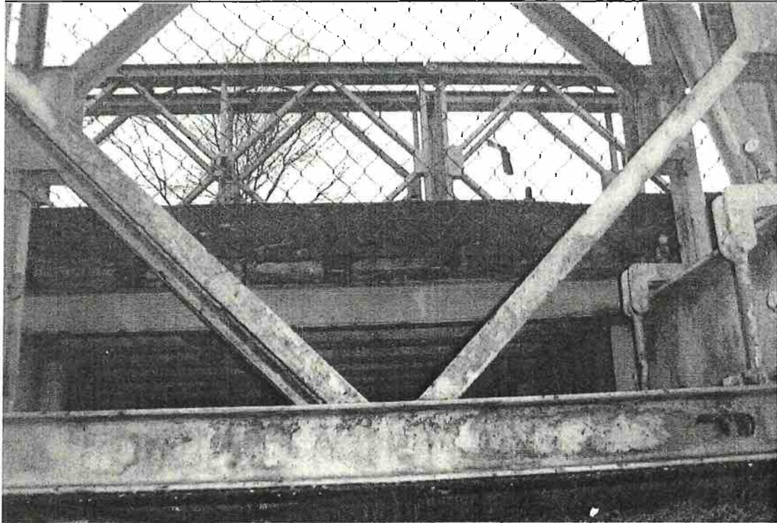
Showing horizontal splits in the end of the timber chesses
