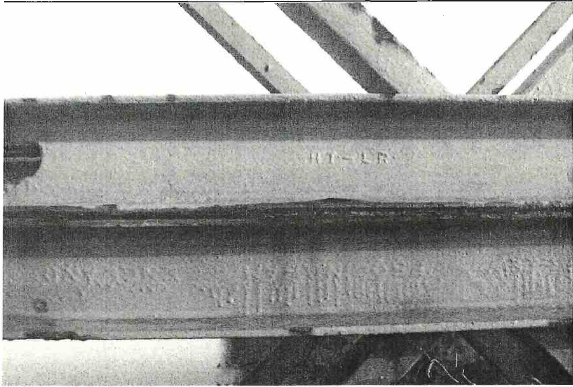
Showing extent of corrosion where the bottom panel meets the top panel.
