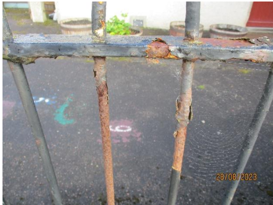
63. Surface corrosion to metal railings
