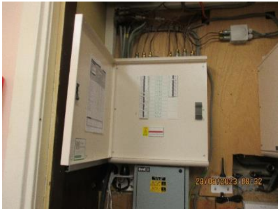
147. Distribution board L+P cupboard 1/19.
