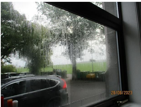
59. Double glazing units fogged with condensation
