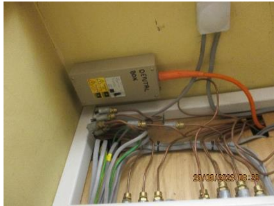
154. RCD unit – dentist box 1/19. (redundant)
