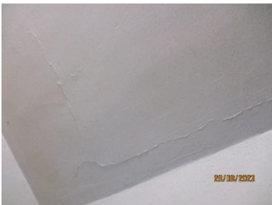
82. Cracking to lath & plaster ceilings
