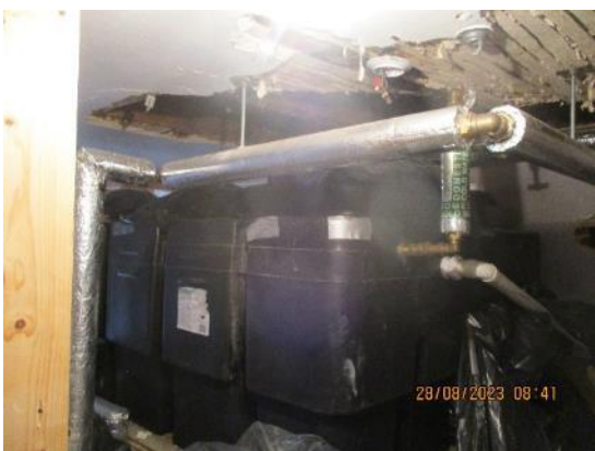
143. Cold water tanks – attic space above 1/7.
