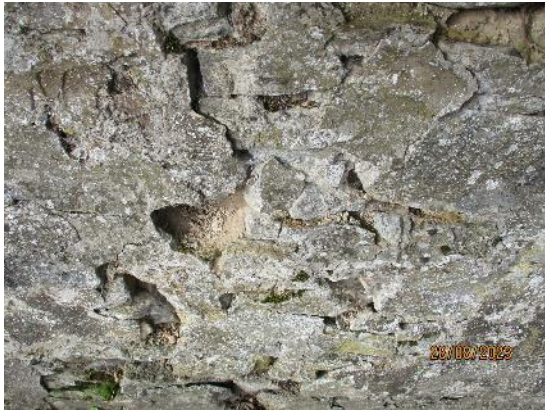
193. Stone wall repairs required
