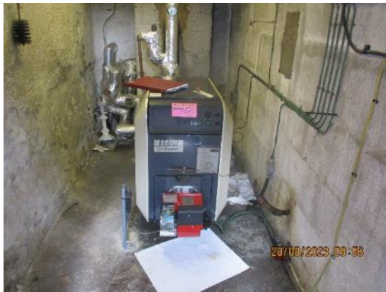
127. Oil system boiler. Basement plant room 0/14.
