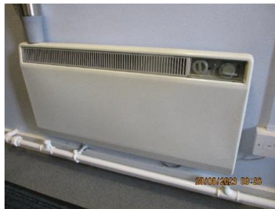
132. Electric convector heater corridor 1/7.
