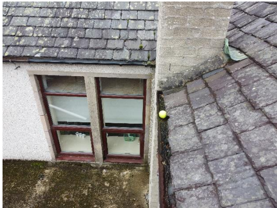
21. Gutters with isolated blockages
