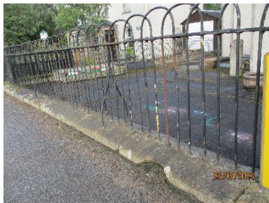
180. Metal hoop fencing
