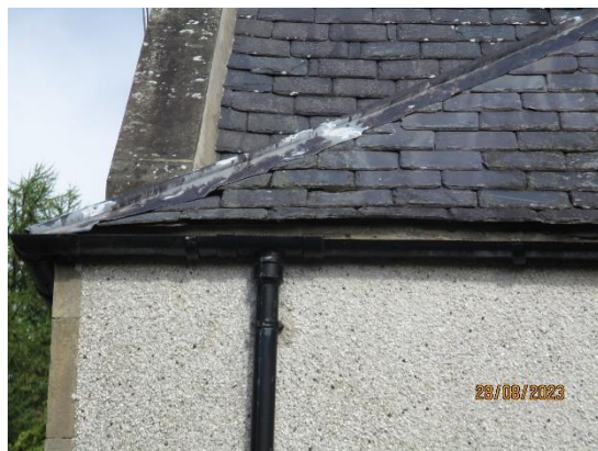
24. Gutter not aligned with roof surface
