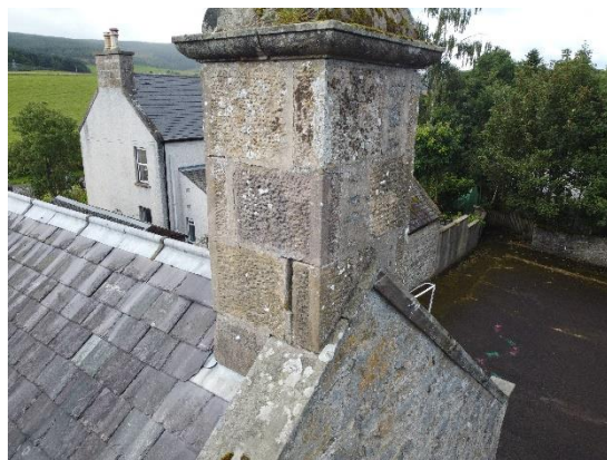
30. Stonework requiring repointing
