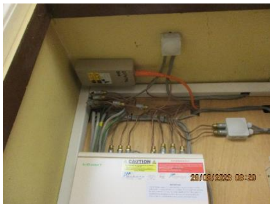
149. General wiring from L+P DB cupboard 1/19.
