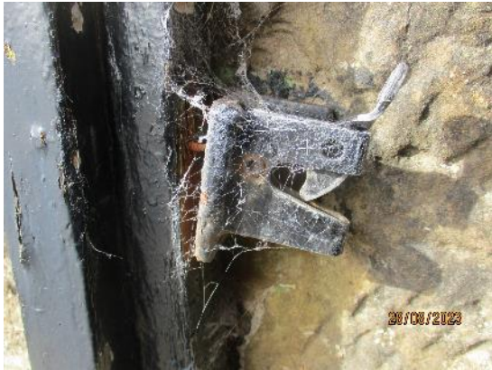
187. Defective damaged gate ironmongery
