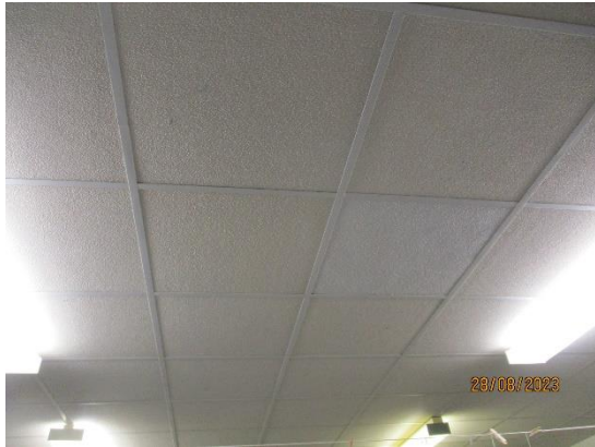
78. Suspended ceiling tiles
