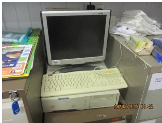
168. CCTV monitor and desktop – office 1/3.
