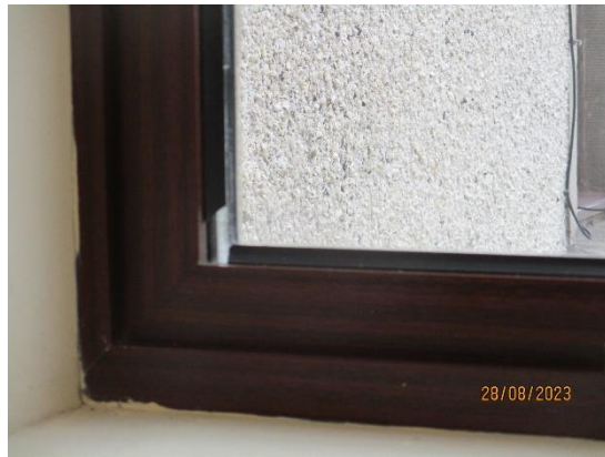
56. Seals failing to double glazed units
