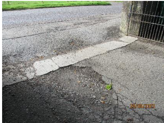
172. Potholes and cracking
