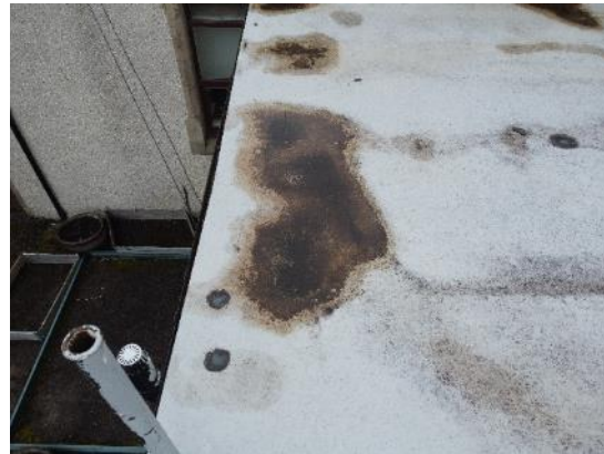
16. Blistered GRP roof with ponding
