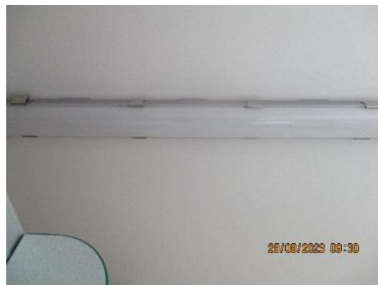
156. Lighting girls toilets 1/9.
