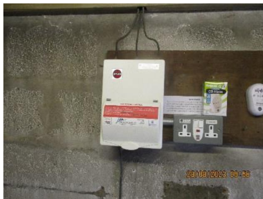
136. Distribution board – heating system. 0/14 supply.
