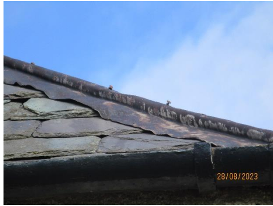
14. Nails protruding from zinc hip
