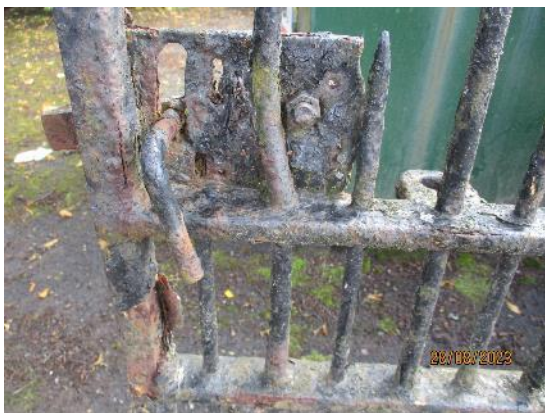
185. Corroded, damaged gates
