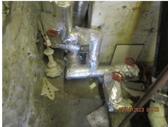
130. Heating system pipework in plant room 0/14.
