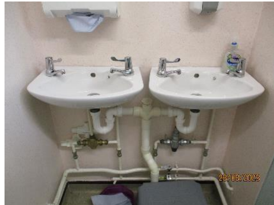
104. Typical wall hung basins
