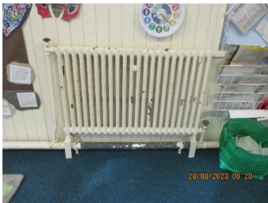
131. Cast iron radiator classroom 1/5.
