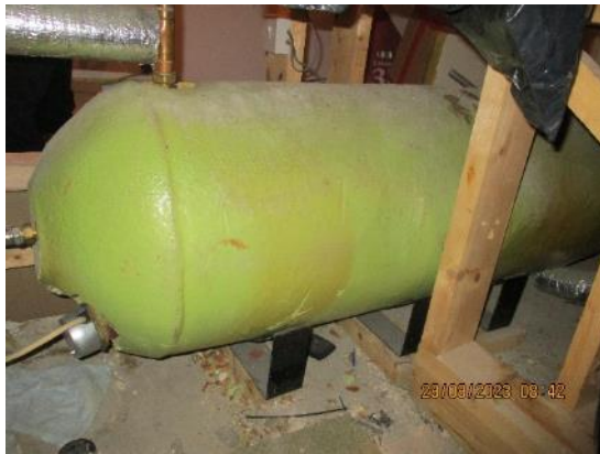
139. Hot water cylinder – attic space above 1/7.
