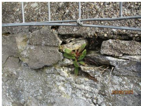
192. Isolated surface erosion
