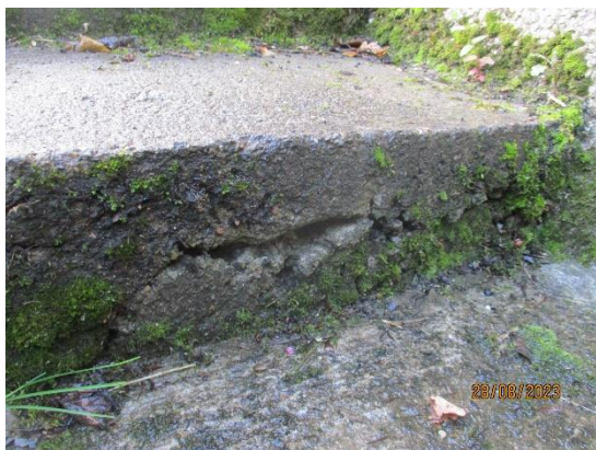
77. Cracked steps to Boiler Room
