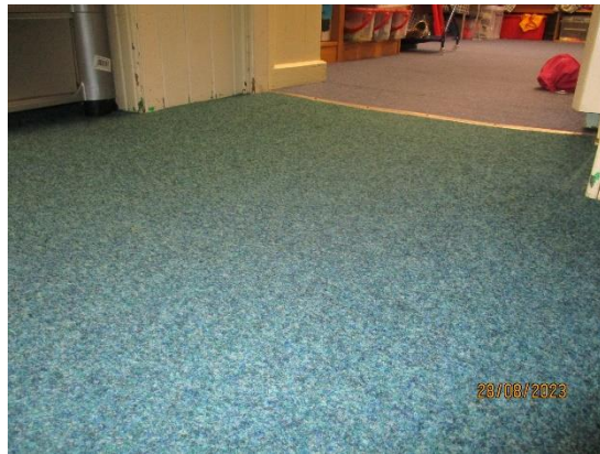
67. Uneven suspended timber floors
