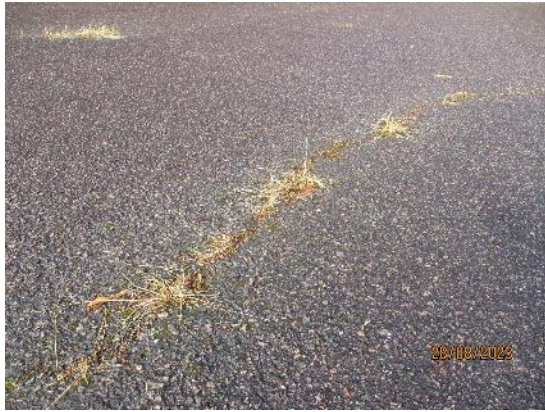
175. Cracked tarmacadam surface
