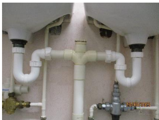
106. PVC waste pipes
