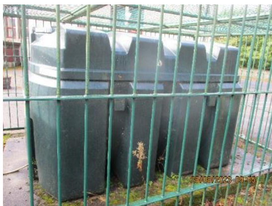
137. External oil storage and supply tank.
