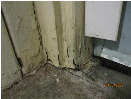
49. Rot in timber doors and frames
