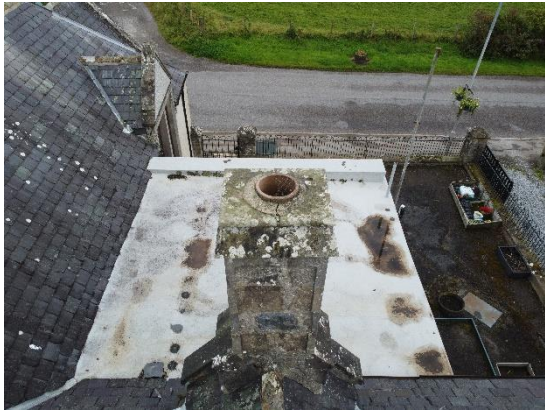
31. Open flues require capping and venting
