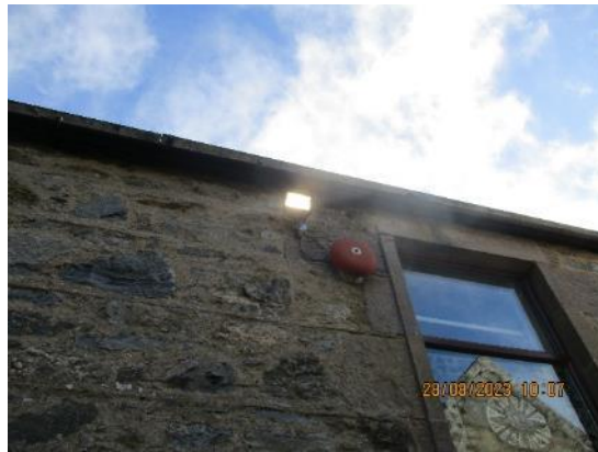
164. External flood light west wall,
