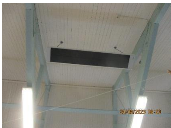
133. Radiant ceiling panel heater classroom 1/6.
