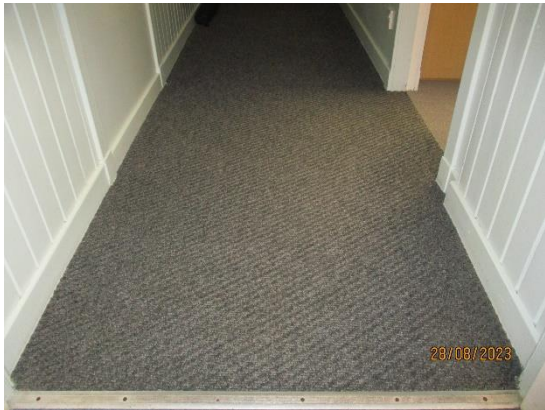
74. Heavy duty carpet to entrance corridor
