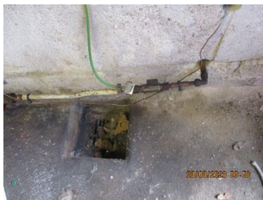
138. Oil supply pipe to appliance 0/14.
