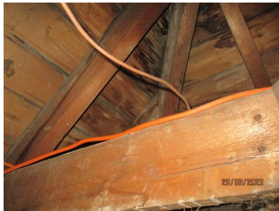
4. Evidence of rainwater penetration
