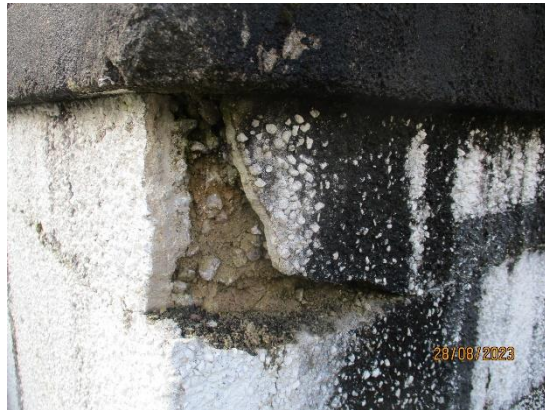
46. Damaged roughcast to Boiler Room
