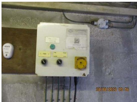
135. Heating control panel 0/14.
