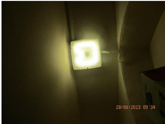
159. Lighting staff toilet 1/11.
