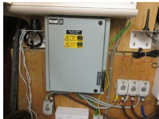
150. Fused isolator cupboard 1/19.
