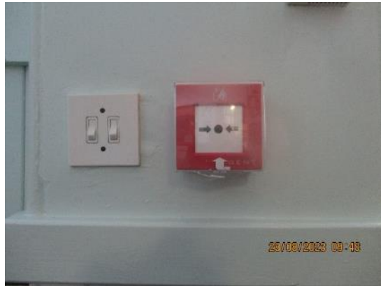
166. Fire alarm call point 1/1.
