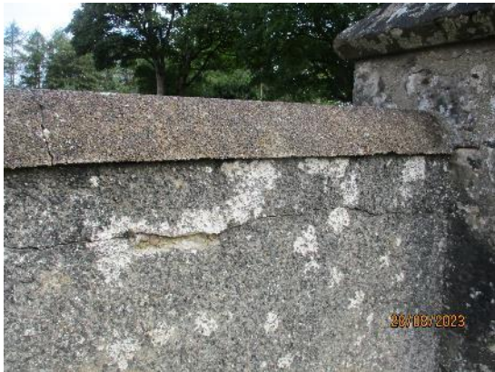
195. Cracks and spalling roughcast
