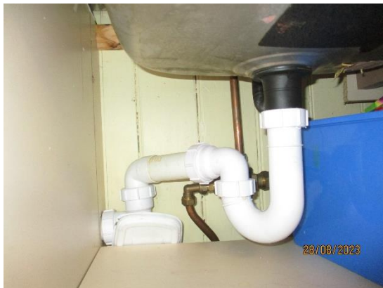
115. PVC waste pipes
