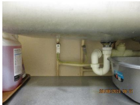
142. Hot water pipework typical.
