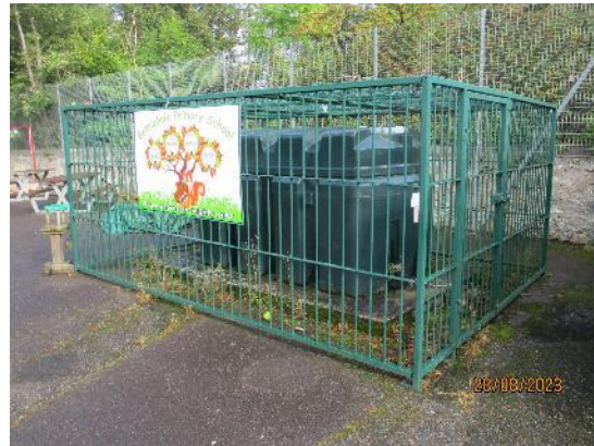
202.Oil tank enclosure
