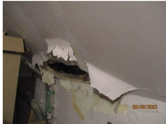
81. Damaged plaster in isolated areas
