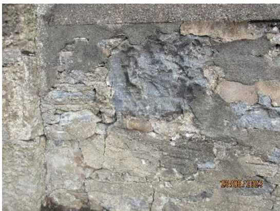
191. Isolated cracking, pointing required
