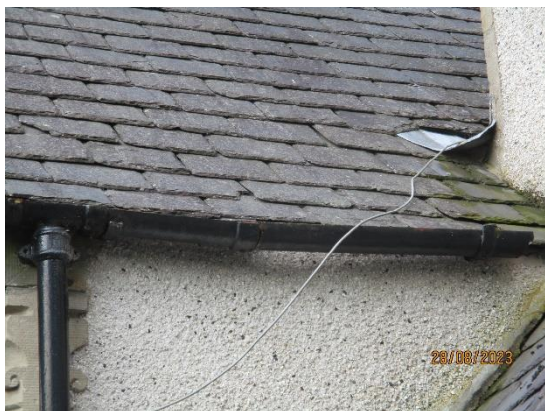
23. Sagging cast iron gutter
