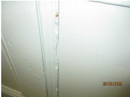
91. Surface damage to doors
