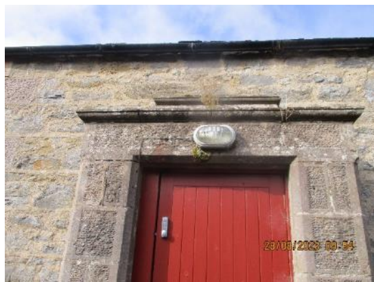
162. External lighting east wall.
