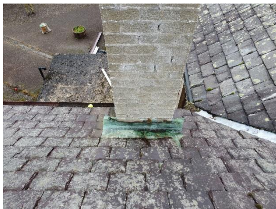
35. Defective flashing to boiler flue
