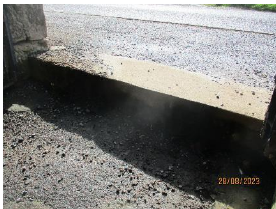
179. Cracked concrete step at entrance
