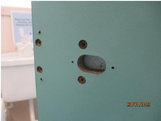
109. Defective and replacement latch mechanism
