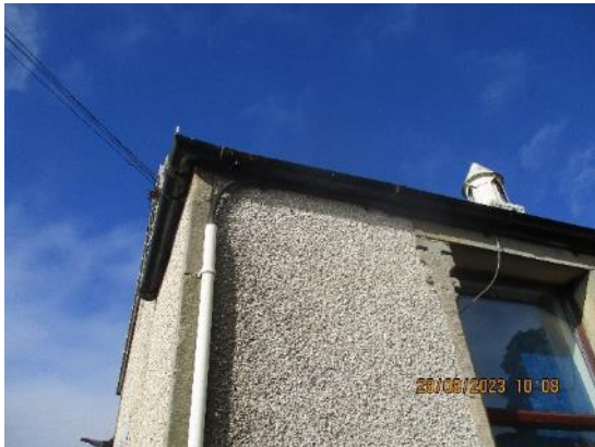
153. Incoming power supply in white PVC pipe.
