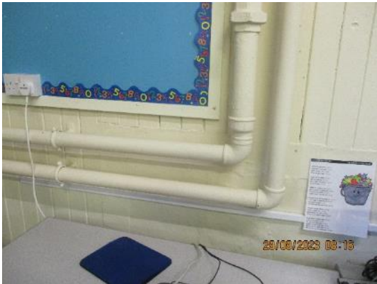
129. Heating system distribution pipework class 1/6.
