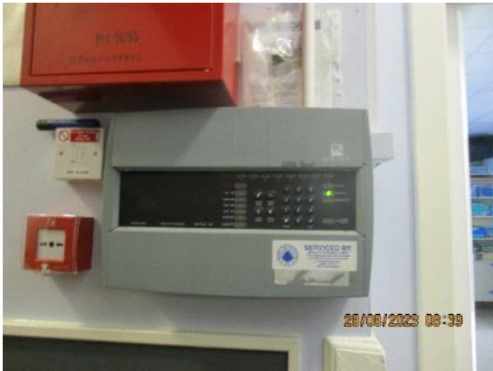
165. Fire alarm system control panel 1/7.
