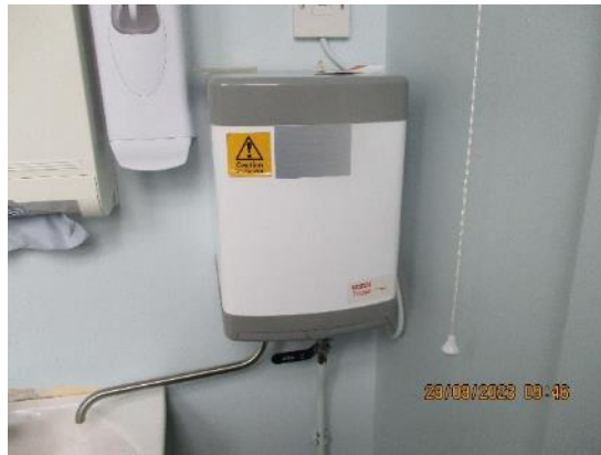
140. Electric point of use water heater 1/2 toilet.
