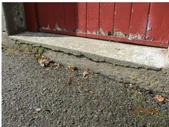
65. Spalling render to concrete steps
