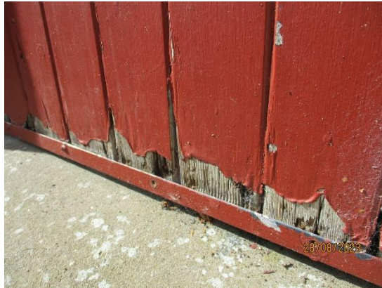
62. Peeling paint to timber doors
