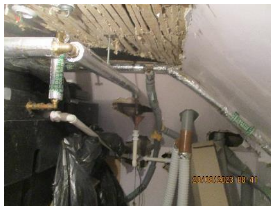
144. Cold water pipework attic above 1/7.
