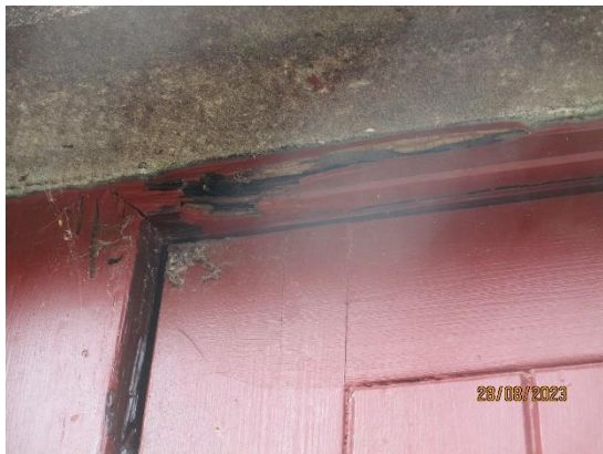
52. Extensive wet rot in timber frames
