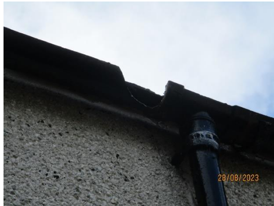
22. Broken section of cast iron gutter
