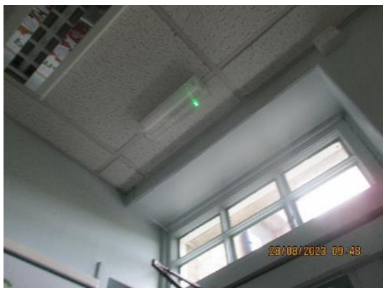
161. Emergency lighting main entrance 1/1.
