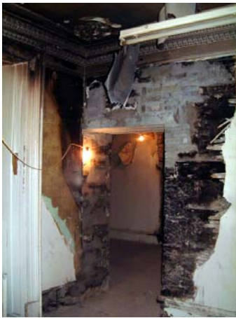
Fire damage to the wall between the boudoir and former Morning Room
