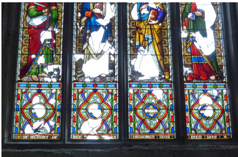
Vandalised stained glass at the Castlehill Church
