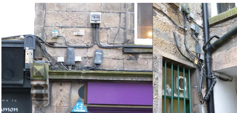
Untidy cables and cable boxes on buildings
