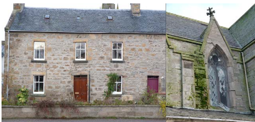
Façade showing distortion in lintels and cills from ground conditions and a gablet at the Castlehill Church showing structural distortion from the failure of an internal beam
