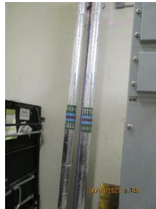
353. Heating pipework main school internal.
