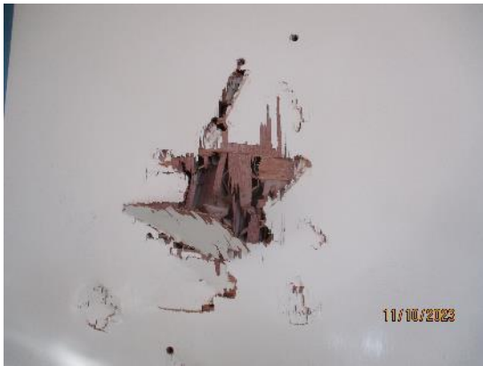
260. Damaged hollow core doors
