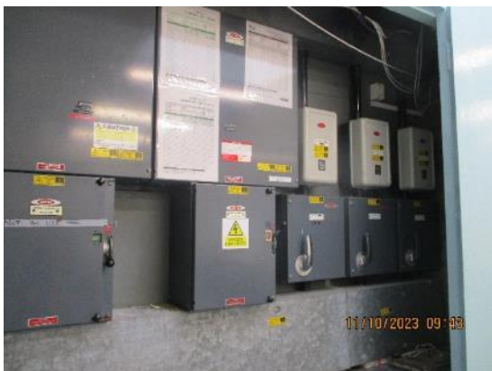
396. Switchgear – kitchen block.
