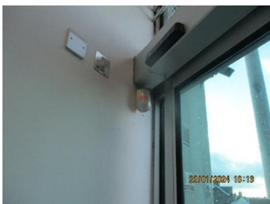
494. Intruder alarm motion sensor main entrance door
