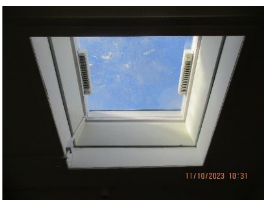
384. Extract fans in roof light K Block.
