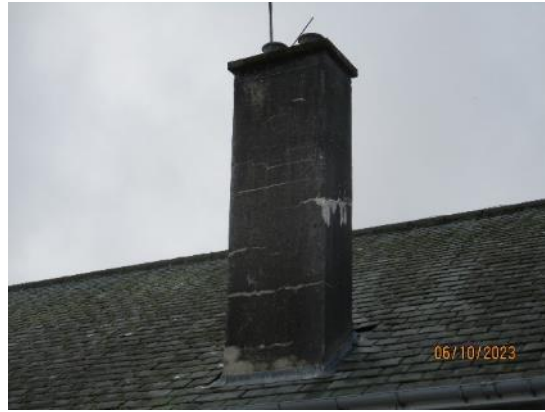
74. Roughcast finish is cracked
