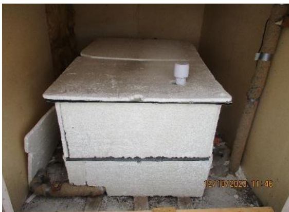
372. Cold water pipework M block tank room.
