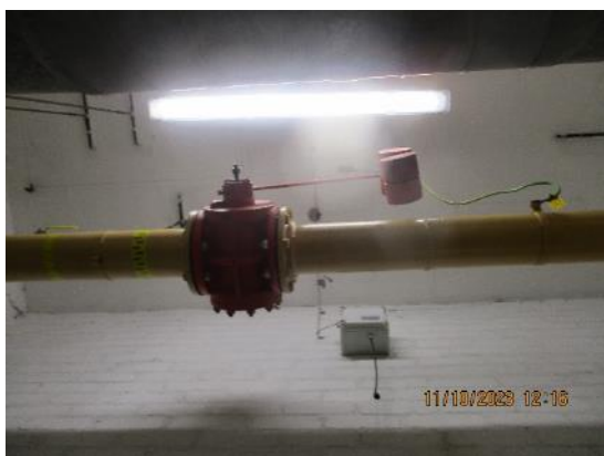
374. Gas supply pipework entering plant room with weighted drop isolation valve.
