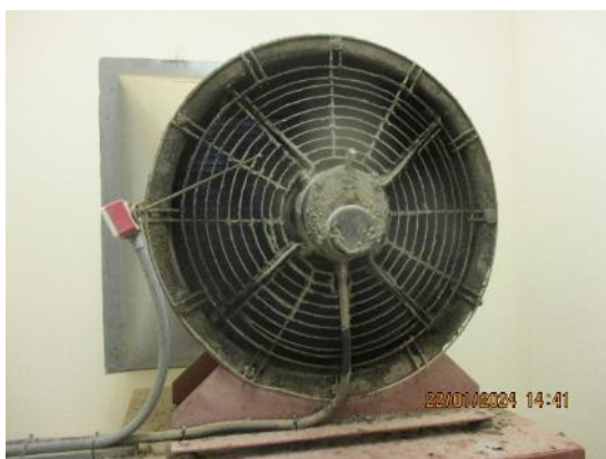
474. Extract fan for pool hall in service duct under pool.
