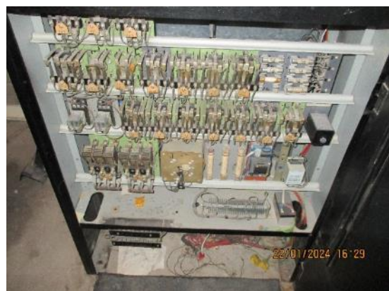
505. Lift electronic control panel.
