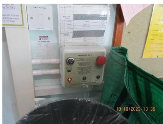
379. Gas safety room control panel typical.
