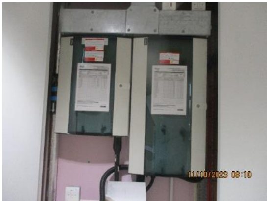
400. Distribution boards – Art dept main school.
