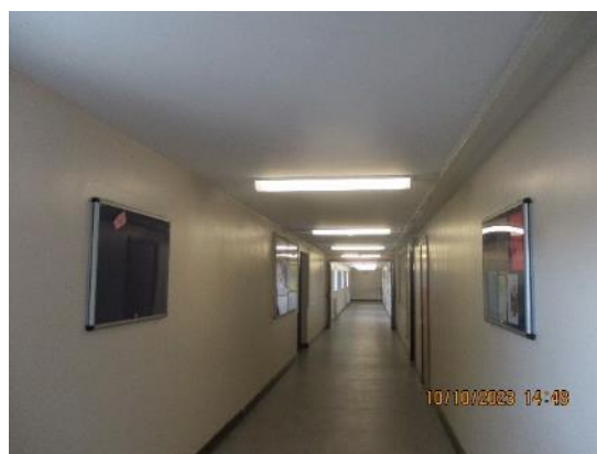
413. Lighting – upstairs corridor main school.
