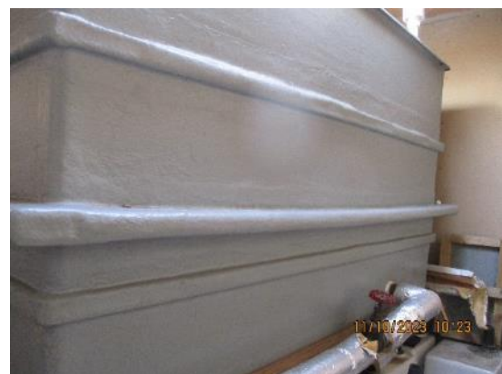
367. Cold water tank K Block
