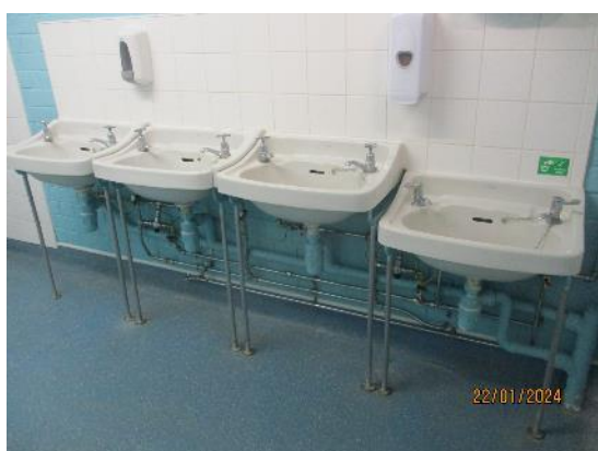
293. China hall hung basins – Leisure Centre
