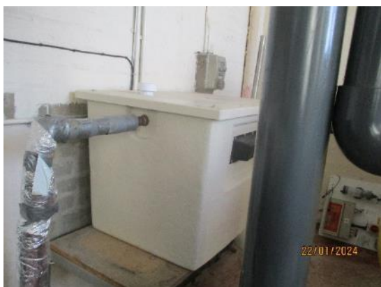
458. Cold water storage tank – pool systems top up.
