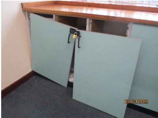
342. Collapsing base units
