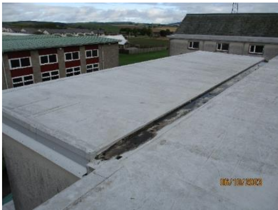
57. SPM box gutters need cleaning
