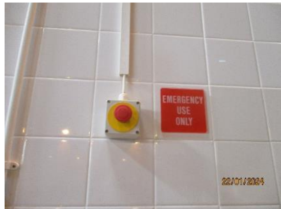
503. Emergency alarm system push button – pool.
