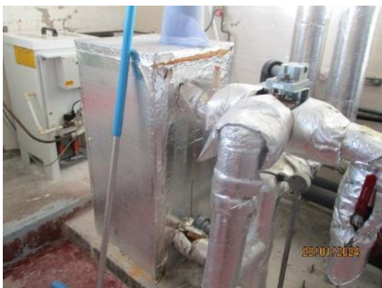
450. Heating pipework and pool plate heat exchanger
