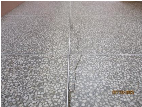
157. Terrazzo tile with isolated damage
