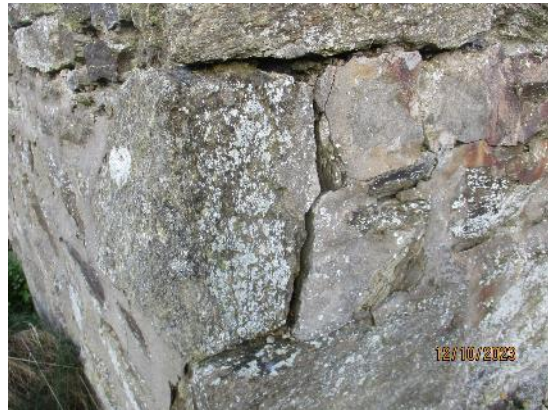
539. Loose stones and repointing required
