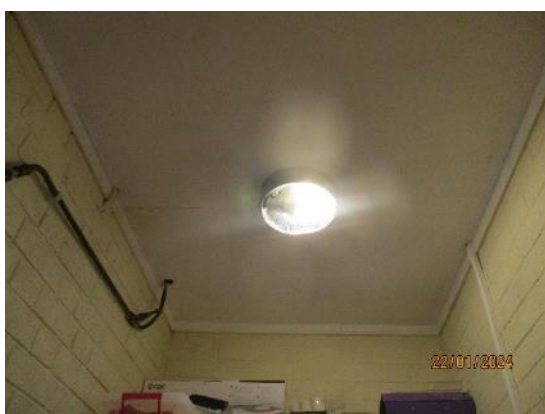
488. Lighting – stores typical
