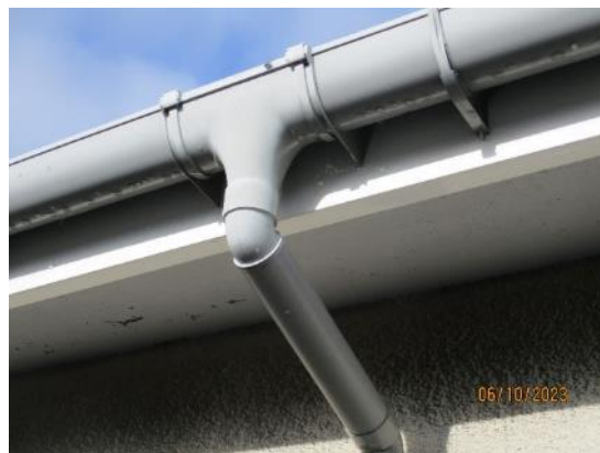
66. UPVC downpipes - School
