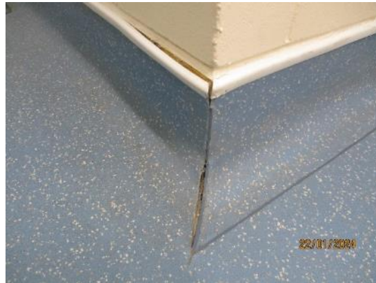
169. Peeling skirting and open joints
