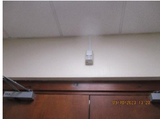
429. Intruder alarm PIR typical.
