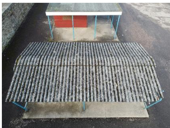
17. Asbestos roofs to Store and Cycle Shelter
