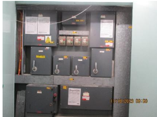
395. Switchgear and busbar – K Block.
