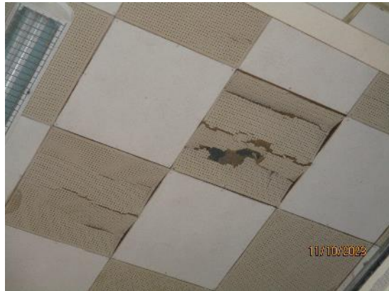
203. Damaged fibre ceiling tiles
