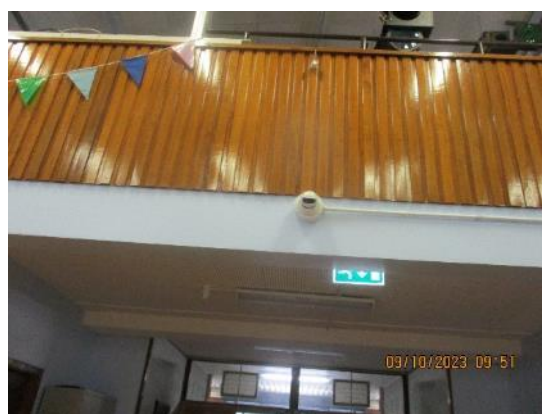
441. CCTV camera assembly hall main building.
