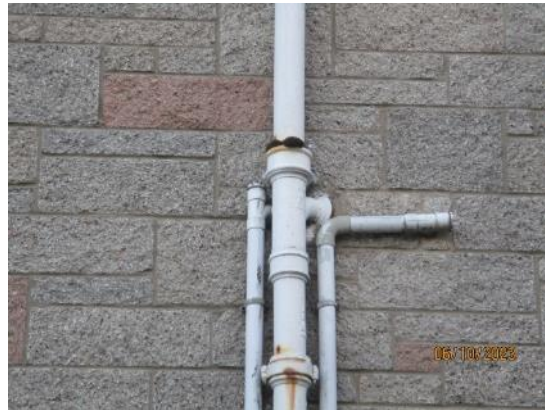
64. Cast iron downpipes leaking - School
