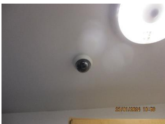
496. CCTV camera typical
