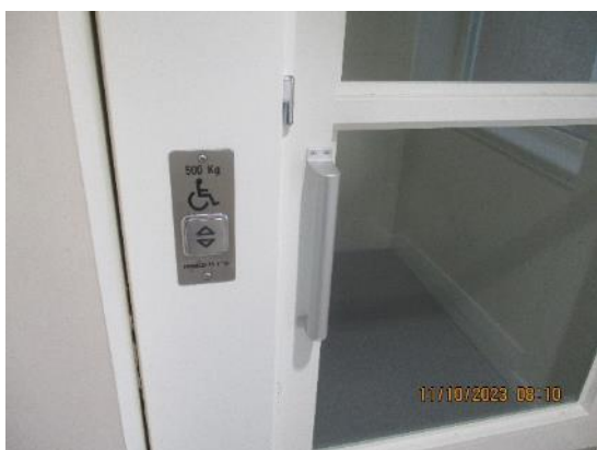
436. Platform lift 2 – front view.
