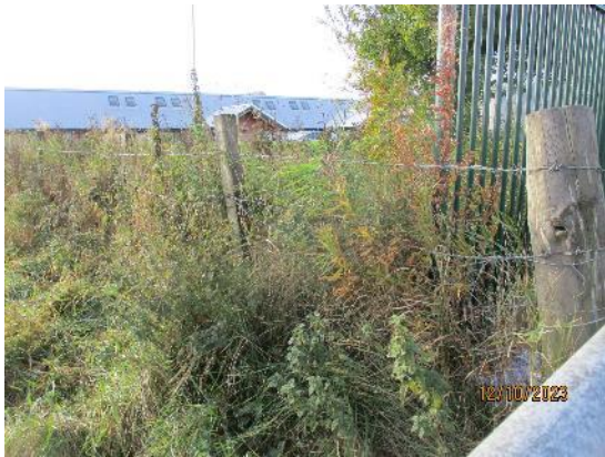
530. Timber post and rail fence leaning
