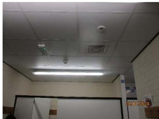
487. Lighting ladies toilets
