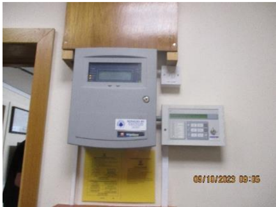
422. Fire alarm control panel 1/2 corridor main school.
