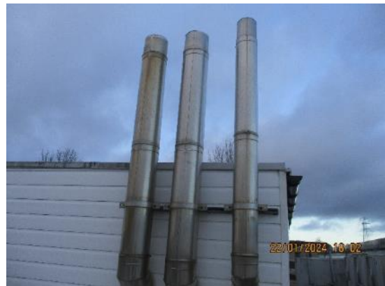
447. Gas boiler flue pipe terminations
