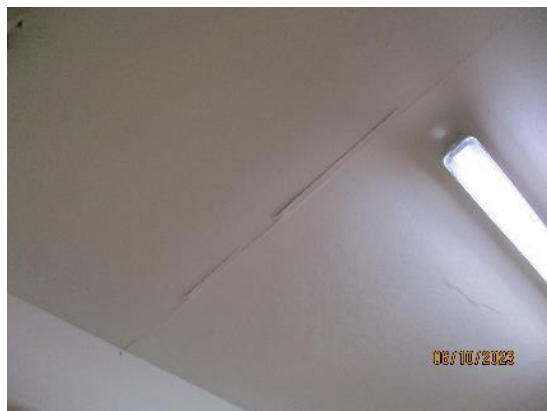
205. Failed taped joints
