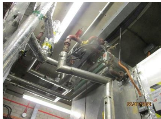
451. Heating pipework plant room 1/7
