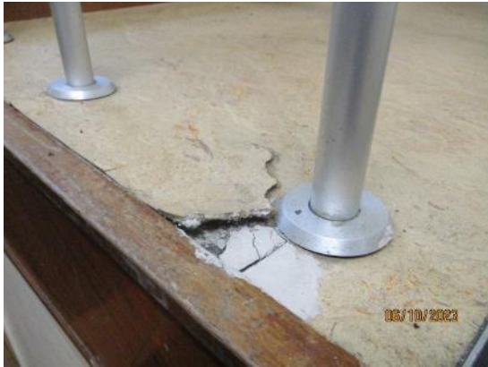
184. Damage around guard rails
