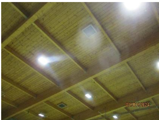
486. Lighting – sports hall
