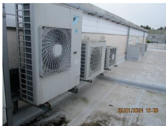
467. Air conditioning external units on roof.
