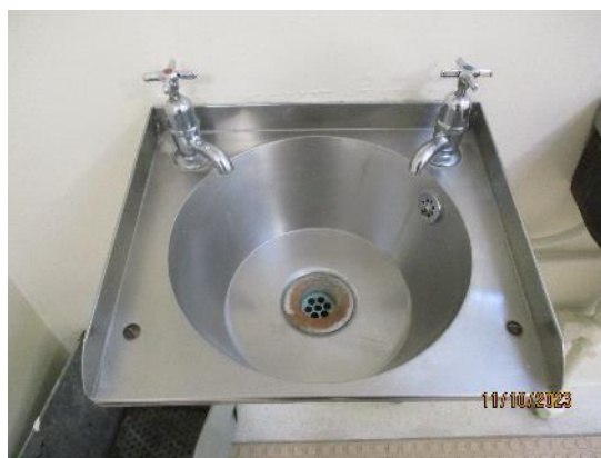
290. Stainless steel wall hung basin – Changing Room
