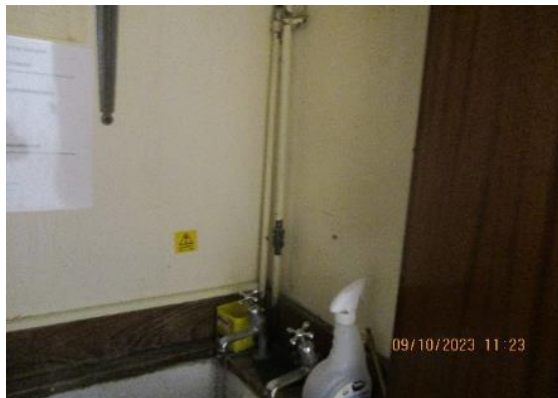
364. Hot water copper pipework main school.
