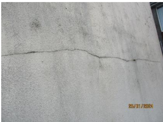
89. Cracks in roughcast
