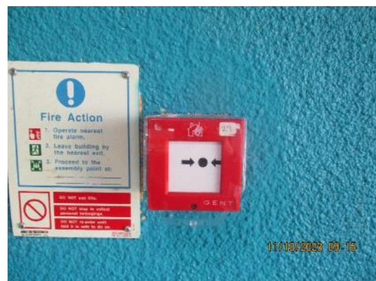
427. Fire alarm call point K block.
