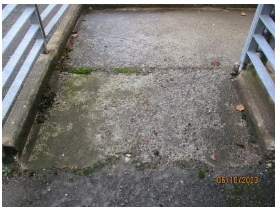
141. Surface erosion of concrete ramps
