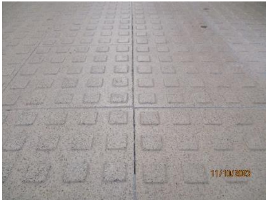
162. Isolated re-grouting required
