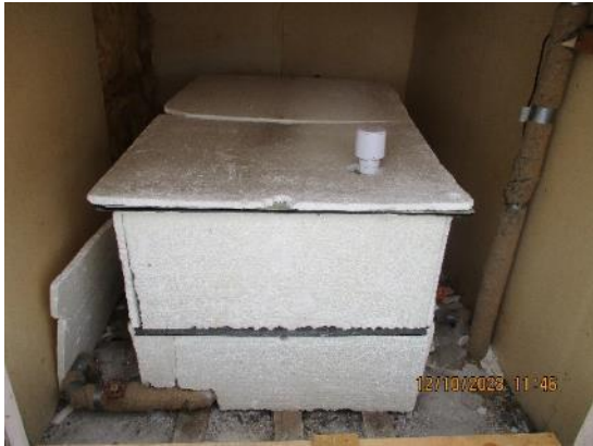
368. Cold water tank – M Block roof.
