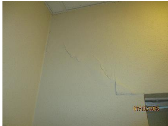
227. Cracked plasterboard walls
