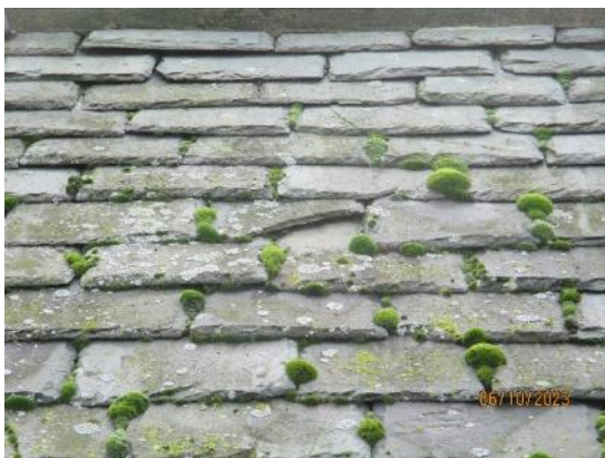
11. Slipped and broken slates
