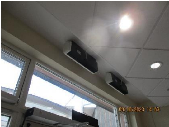
356. Electric fan over door heaters main school.
