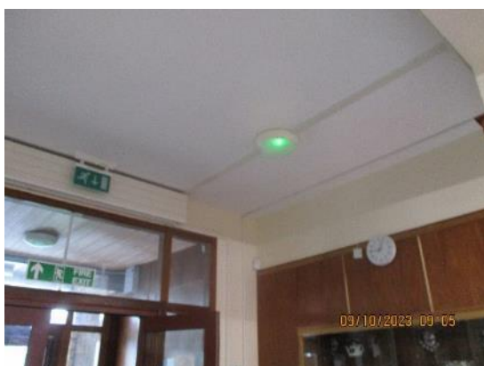
418. Emergency lighting main school.
