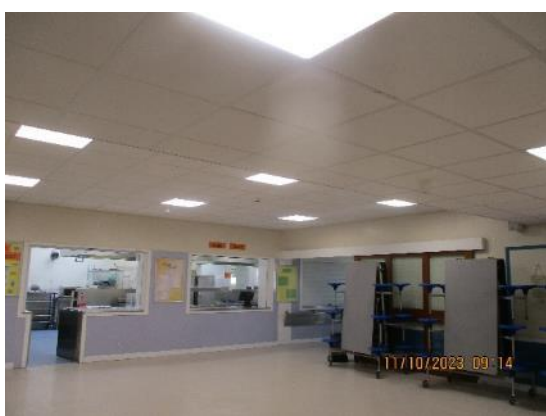
414. Lighting – K Block dining room.
