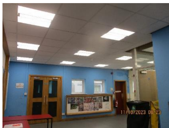
419. Lighting incorporating emergency fittings K Block upstairs.
