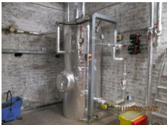
360. Hot water storage calorifier main school.
