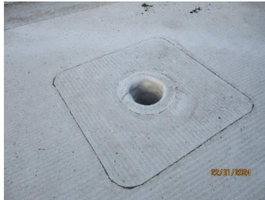
70. Internal downpipes missing balloon gratings
