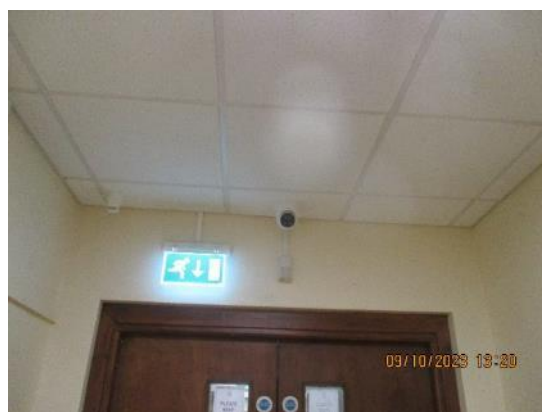
443. CCTV camera internal corridor main building.
