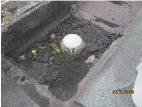
61. Felt box gutters blocked – Leisure Centre
