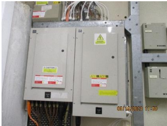
398. Distribution boards – Main school typical
