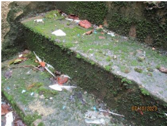
137. Isolated damage to concrete steps
