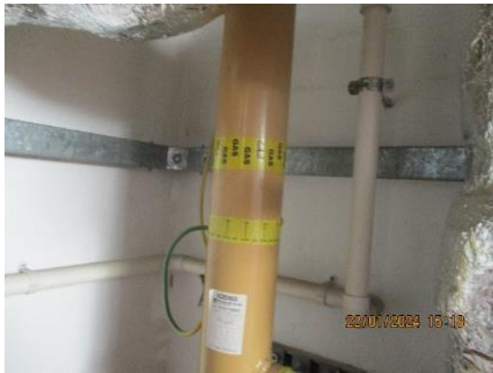
476. Gas supply pipework in boiler house.
