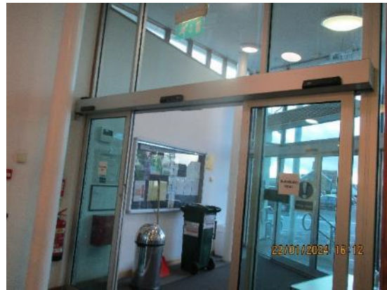
501. Electronic automatic doors reception entrance lobby
