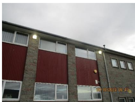
421. External lighting main school building.
