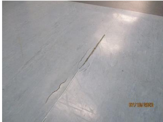
150. Cracked and damaged sheet vinyl
