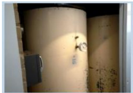
361. Hot water calorifiers kitchen block
