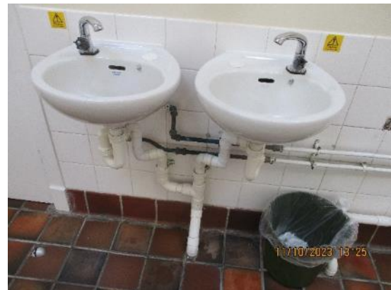
365. Hot water copper pipework M Block typical.
