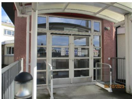
103. PVC electric doors - School
