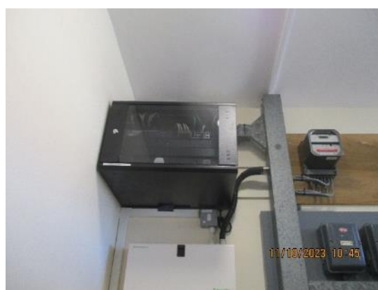
439. CCTV distribution cabinet – K block
