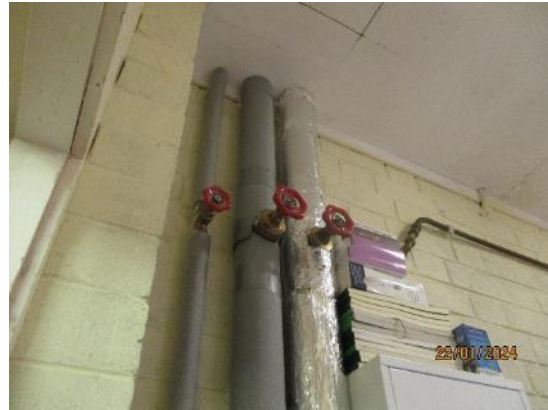
453. Hot water pipework - typical
