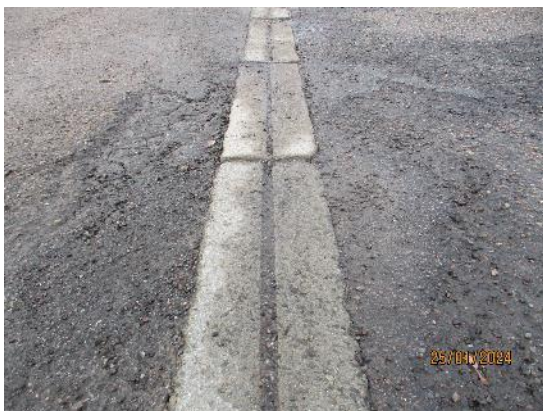
546. Channel gullies blocked – Leisure Centre
