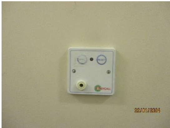
500. Disabled toilet alarm system device – typical.
