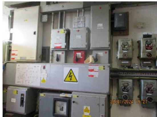
479. Switchgear – boiler house 1/S22
