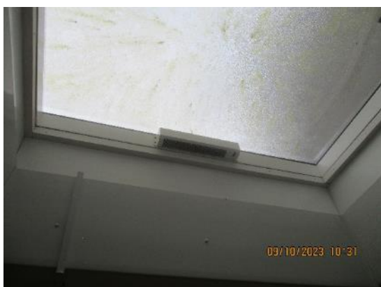
382. Extract fan in rooflight typical – main school.
