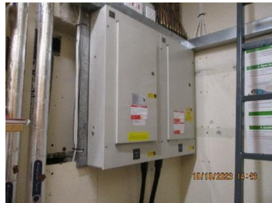
401. Distribution boards – science dept main school.
