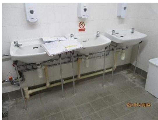
465. Cold water distribution pipework typical.
