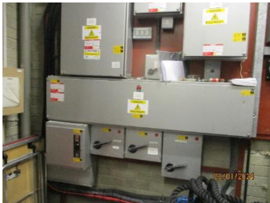
478. Switchgear – plant room 1/7
