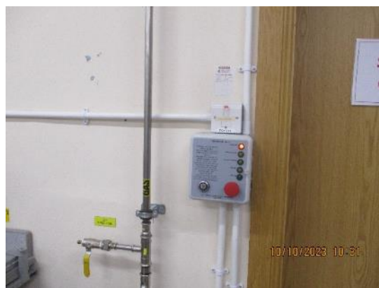
381. Gas safety control panel technology class.
