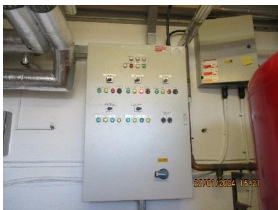
456. Control panel – boilers and pumps
