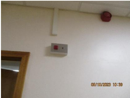
430. Disabled toilet alarm alert unit. 1/76 Toilet
