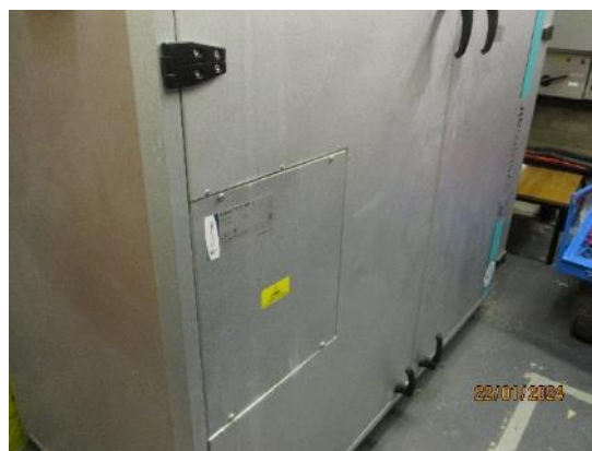
469. AHU – heat recovery plant room 1/7
