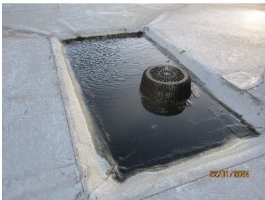
71. Internal downpipes part blocked
