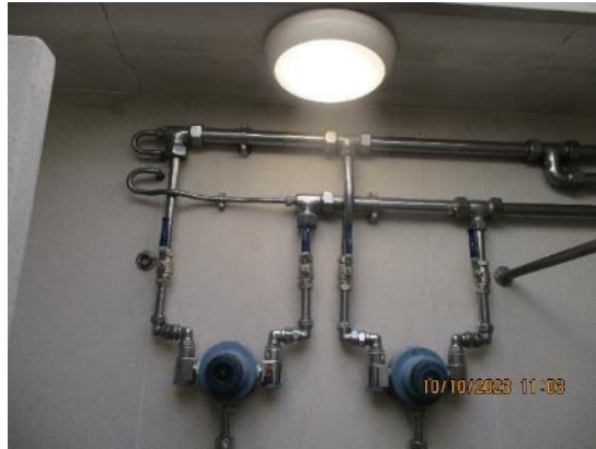
369. Cold water pipework Main school
