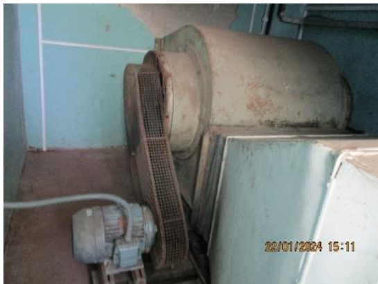
472. Pool hall air handling unit 1/S21
