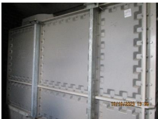
366. Cold water tanks main school.
