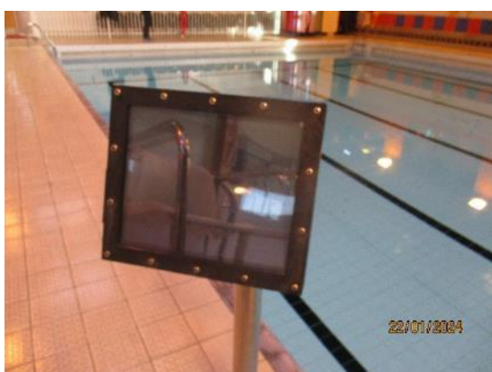
498. CCTV system underwater in pool. - Monitor
