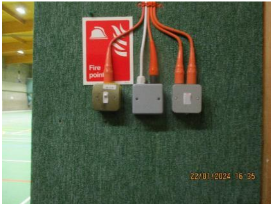
484. Switches – sports hall store
