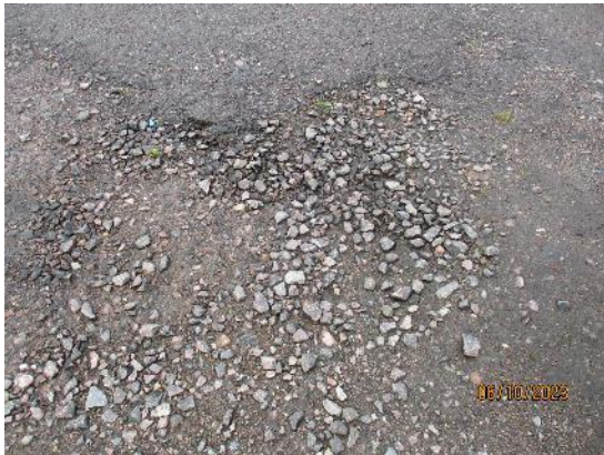
508. Tarmac surface erosion
