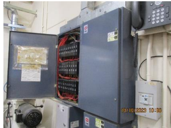
399. Distribution boards – woodwork class main school.
