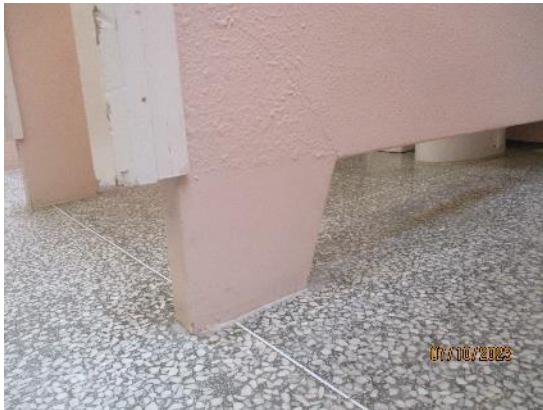
220. Cracking at the feet
