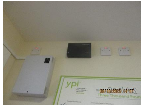
425. Fire alarm interface for reception security door.
