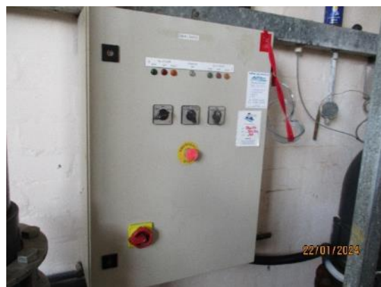
457. Control panel – pool pumps.
