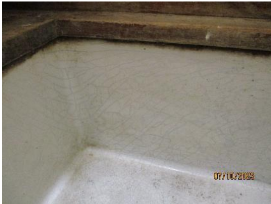
315. Surface crazed and cracked
