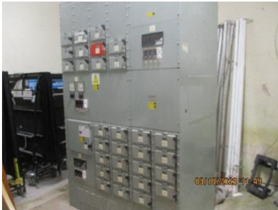
394. Main switchboard – incomer main school 1/67
