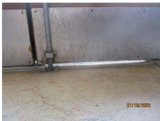
102. Gaps around external doors
