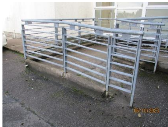
142. Galvanised tubular guard rails
