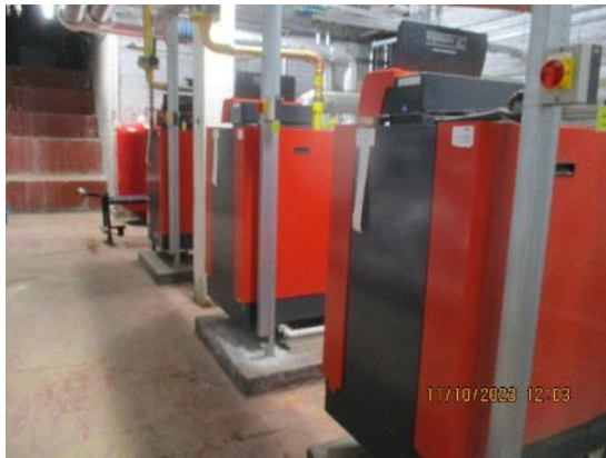
350. 3 no. natural gas fired boilers.
