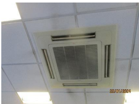
466. Air conditioning unit fitness room.
