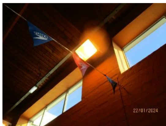
491. Lighting – pool hall
