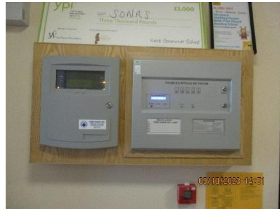
423. Fire alarm control panel new reception corridor.
