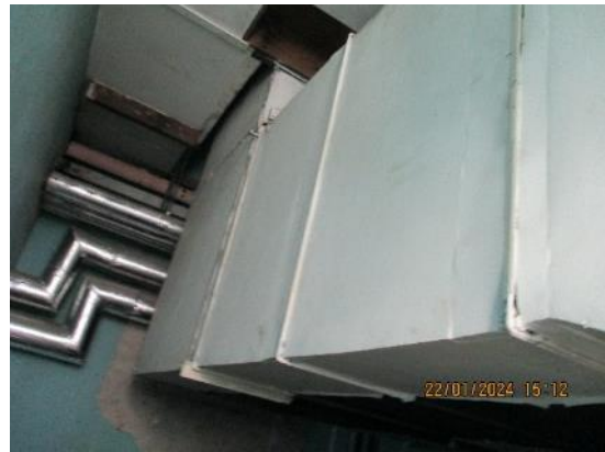
471. Air handling unit ductwork 1/S21
