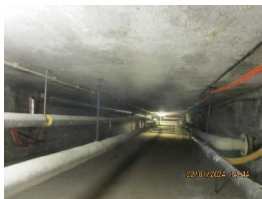
461. Pipework in service duct under pool.
