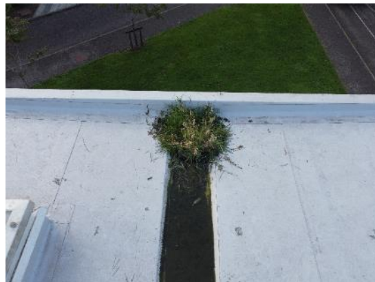
58. Box gutters and outlets blocked
