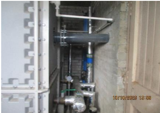
370. Cold water pipework at main school tank.
