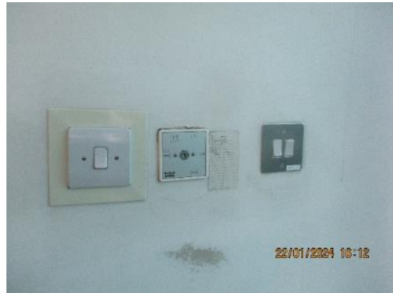
485. Switches – main entrance lobby
