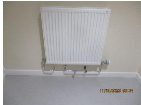
359. Steel panel radiator Main school typical.
