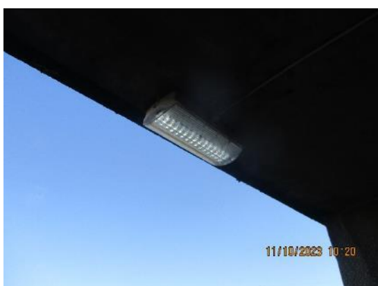
420. External lighting – K block entrance.
