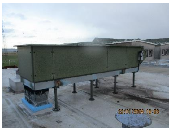
468. Air handling unit on roof.
