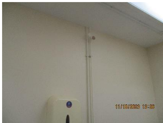
373. Cold water pipework – M Block typical.
