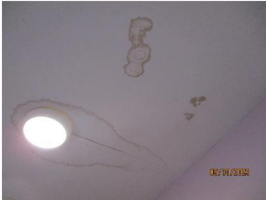
206. Watermarked plasterboard ceilings
