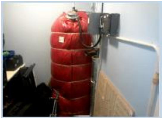
362. Hot water storage cylinder Music block
