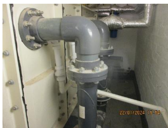
463. Cold water storage tank external view.
