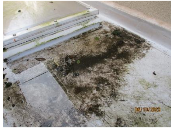
32. SPM roofs ponding
