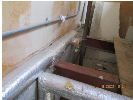
371. Cold water pipework K block tank room.
