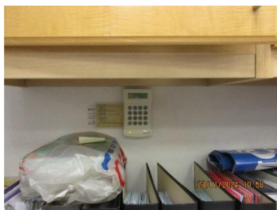
495. Intruder alarm control panel reception
