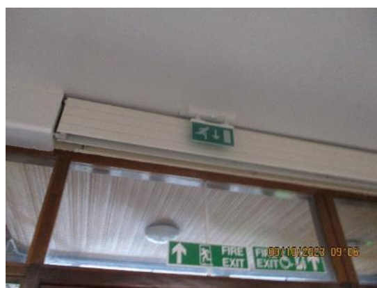
417. Emergency exit lighting main school.
