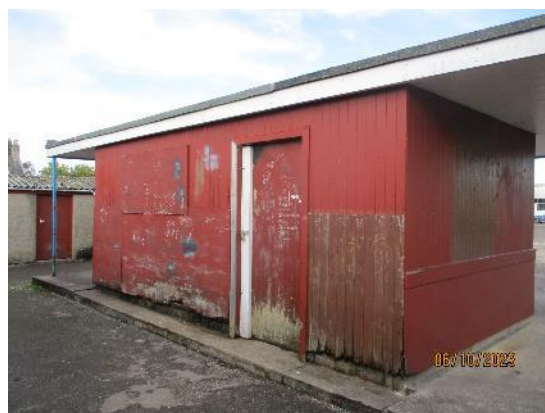
553. Rotten timber linings
