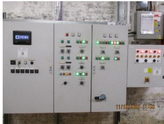
351. BEMS main control panel.
