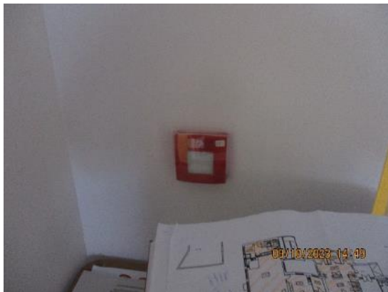
424. Fire alarm call point typical.
