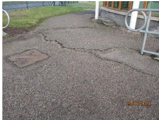
525. Tarmacadam cracked by tree roots
