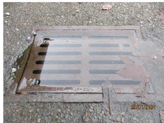
547. Road gullies blocked
