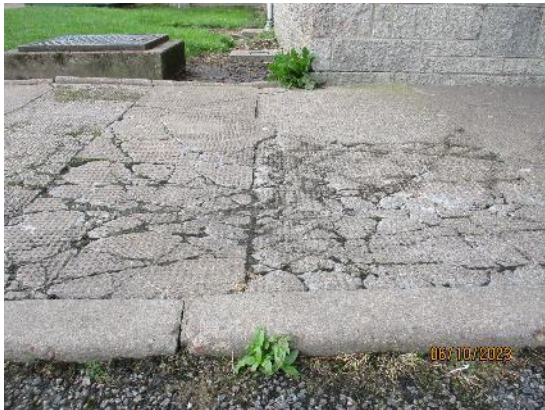
520. Concrete paths sunken
