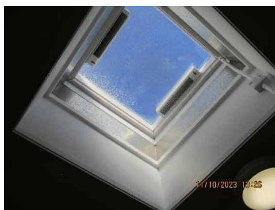
385. Extract fans in rooflights – M block.
