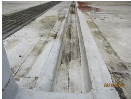
56. SPM box gutters - School
