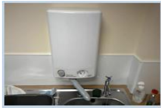
363. Point of use water heater main school.
