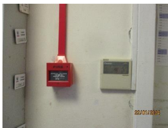
493. Fire alarm call point typical
