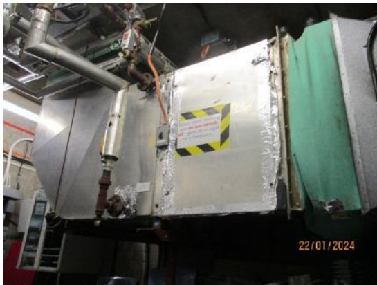
470. Air handling unit plant room 1/7
