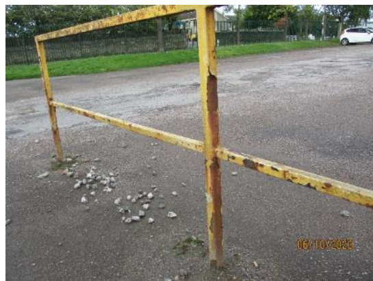
130. Metal separation rails
