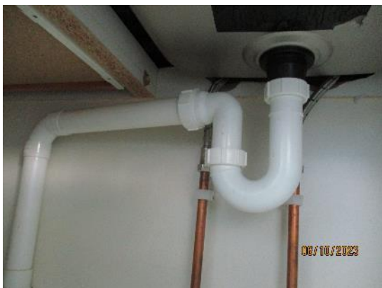
317. UPVC waste pipes
