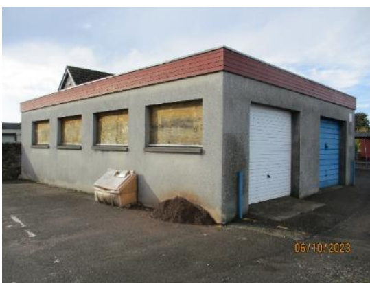
106. Garage up and over doors
