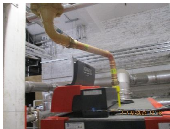
375. Gas supply pipework to boilers.
