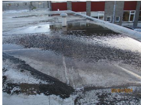
22. Single ply to Leisure Centre - Ponding
