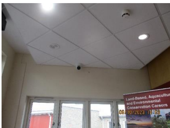
442. CCTV camera ASN dept main building.
