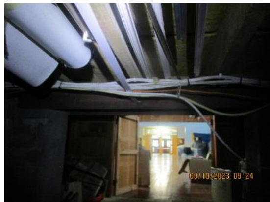
433. General wiring under stage.
