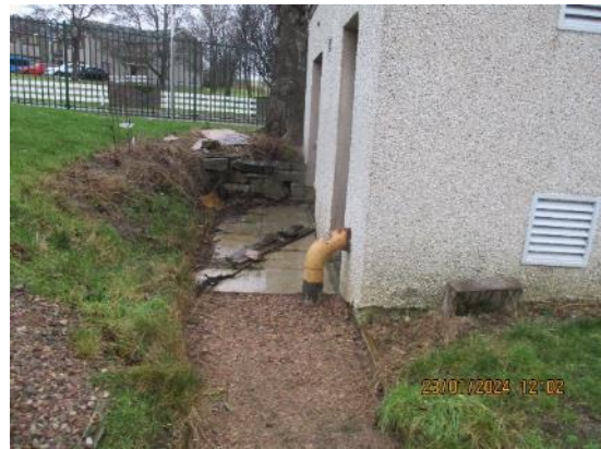
477. Gas meter housing and pipework.
