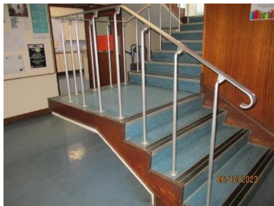
189. Aluminium balustrades - School
