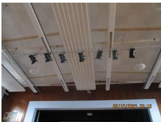
354. Ceiling mounted radiators main assembly hall.
