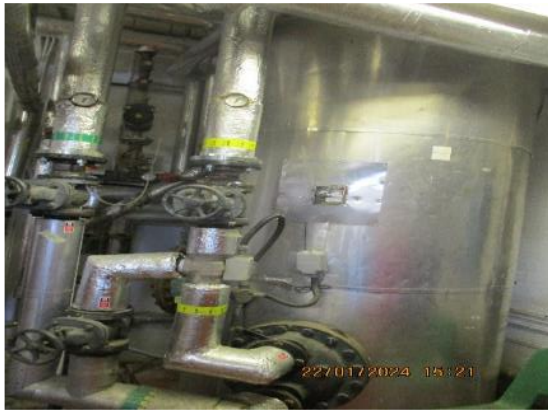
452. Hot water calorifier and pipework
