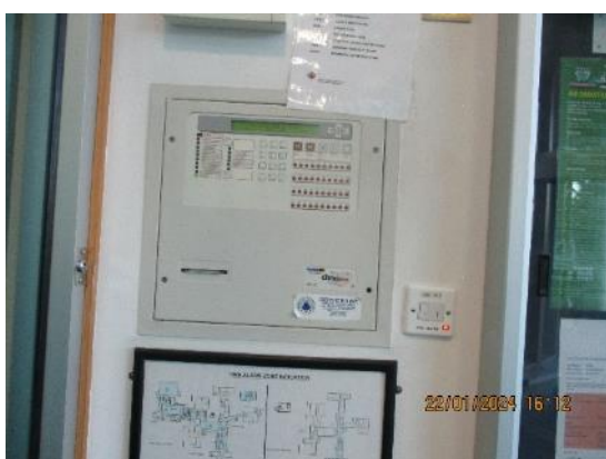
492. Fire alarm control panel entrance lobby
