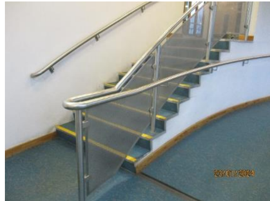
193. Stainless steel handrails – Leisure Centre
