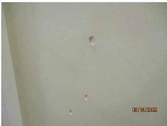
216. Masonry/plaster walls - School
