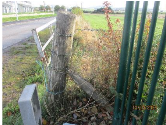
531. Timber strainer leaning
