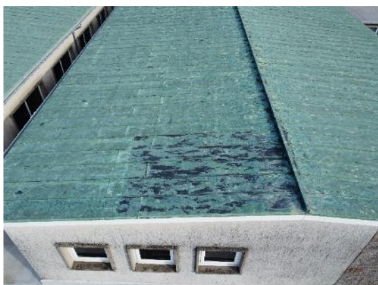
13. Surface discolouration of copper roofs
