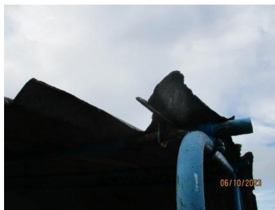
18. Damaged asbestos roofs
