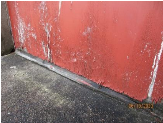
97. Delamination of timber doors
