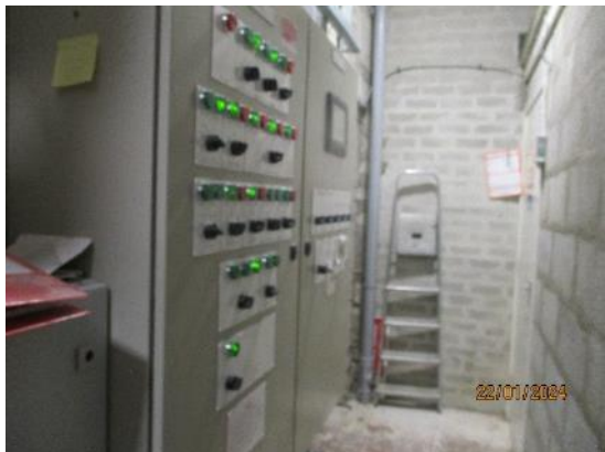
454. Main BMS control panel
