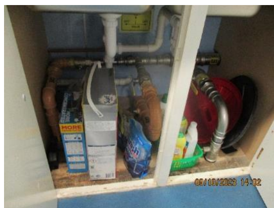
377. Gas pipework entering HE and science departments
