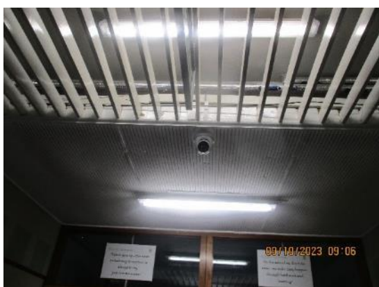
440. CCTV camera entrance lobby main building.
