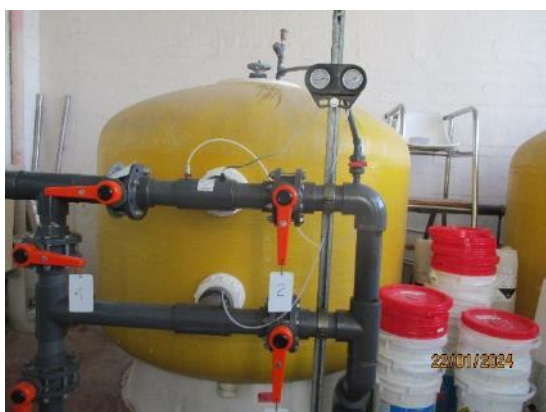
460. Sand filter vessels and pipework – pool systems.
