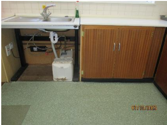
344. Missing base units
