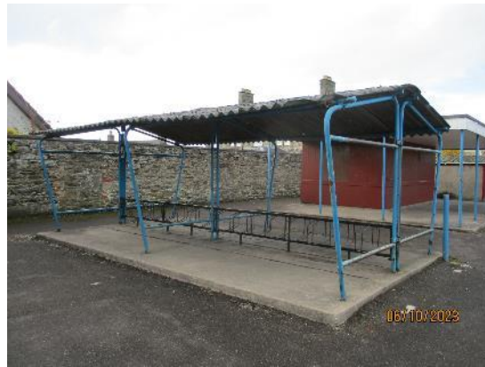
555. Bike shelter with asbestos roof
