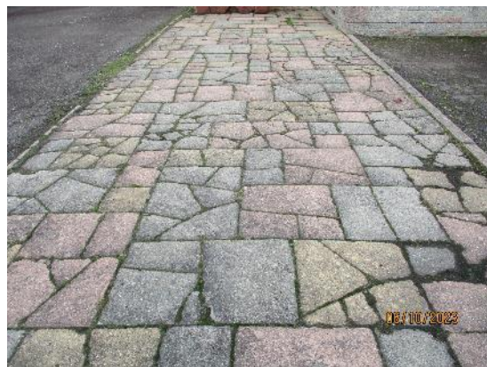
523. Cracked paving slab footpaths
