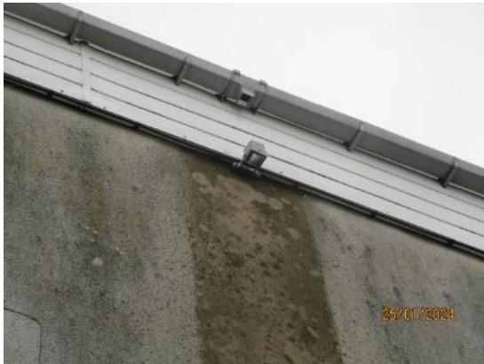
69. Leisure Centre downpipes missing
