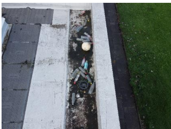
59. Block M – blocked box gutters
