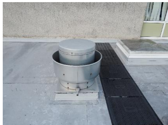
391. Kitchen canopy extract fan – K Block roof.
