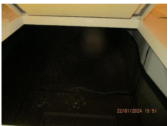
462. Cold water storage tank internal view.
