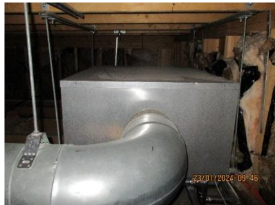
473. Air handling unit above sauna in roof void.
