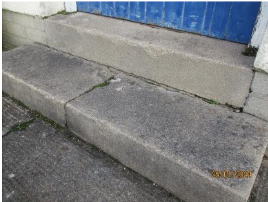
139. Broken concrete steps to plant rooms
