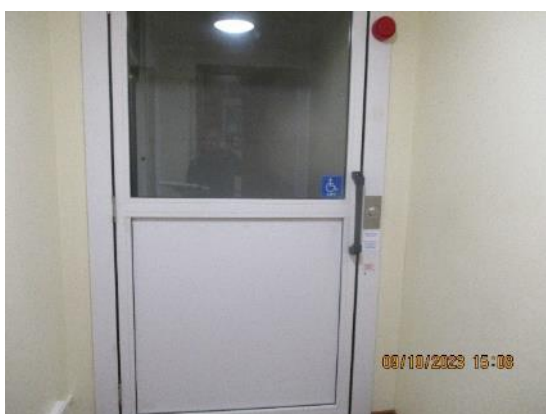
434. Platform lift 1/116 – front view.
