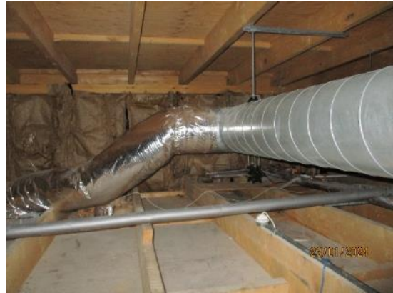
50. Lack of insulation above Sauna
