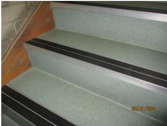
186. Vinyl treads and risers – Leisure Centre
