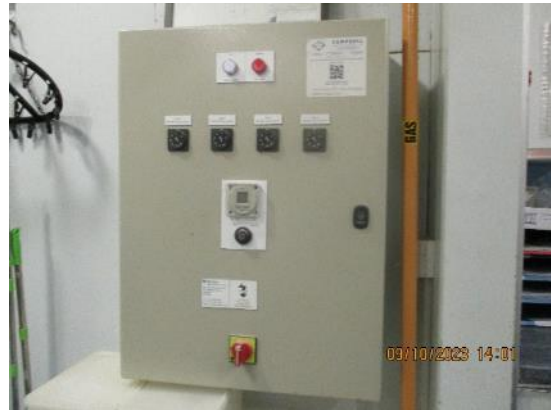
431. BEMS control panel/outstation. Main school.
