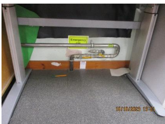
378. Gas supply pipework entering science class.
