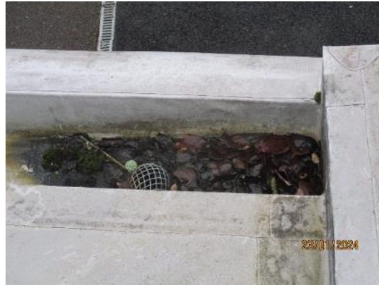
62. SPM box gutters part blocked -Leisure Centre
