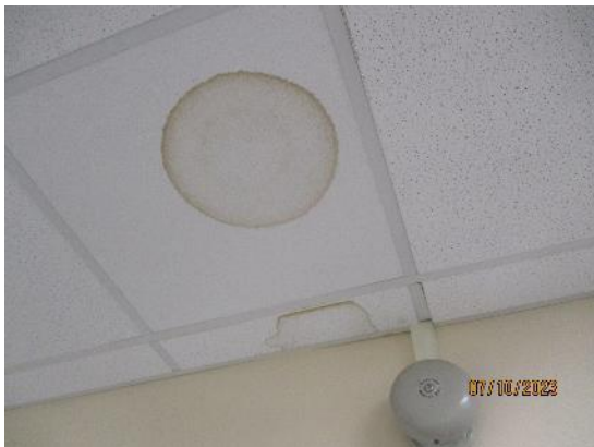
196. Watermarked ceiling tiles
