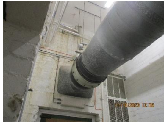
393. Supply fan and ductwork – plant room main school.
