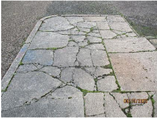
518. Cracked concrete footpaths
