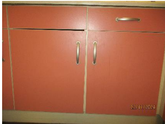
345. Collapsing base units – Leisure Centre
