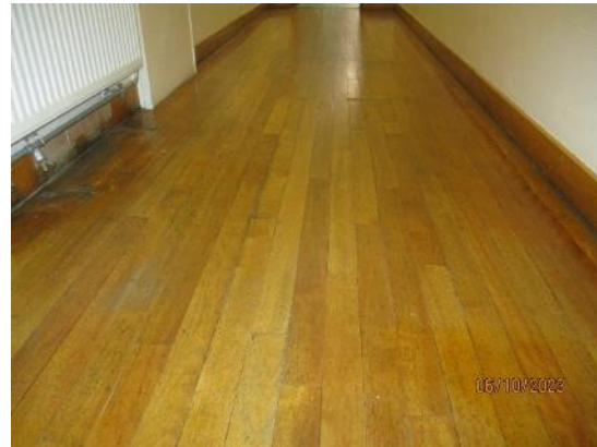
146. Noisy timber floating floors
