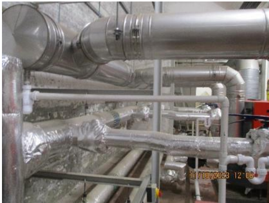
352. Heating system pipework main school plant room.
