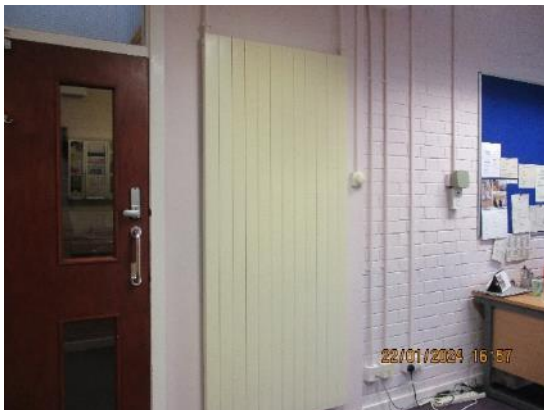
448. Steel panel radiator office 1/4
