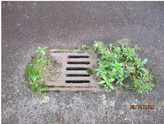
544. Surface water drainage, part blocked
