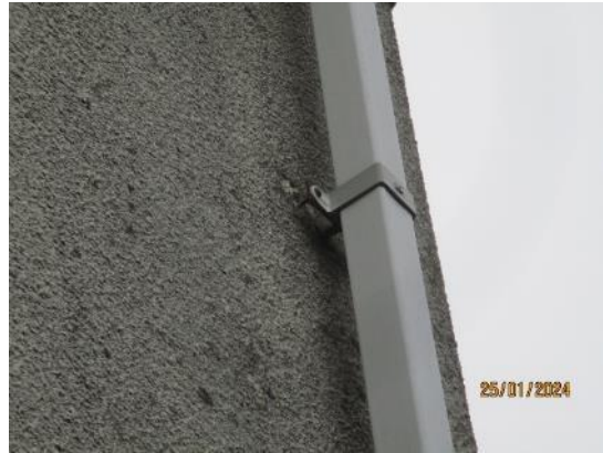
68. UPVC downpipes insecure – Leisure Centre
