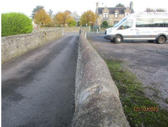
542. Retaining wall to neighbour, leaning
