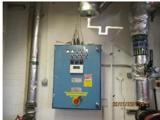
455. Control panel – boiler house
