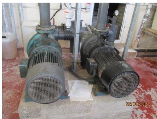
459. Pool system pumps and pipework.
