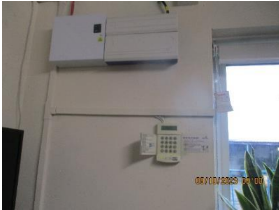
428. Intruder alarm keypad janitors office 1/70
