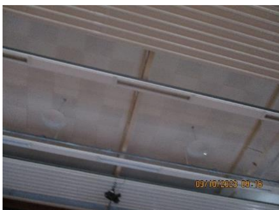
412. Lighting – assembly hall 1/66 main school.
