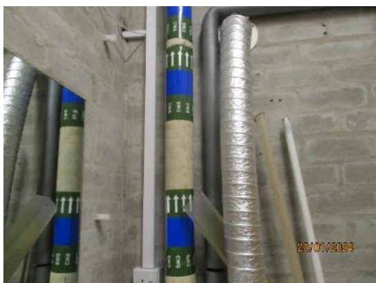
464. Cold water service pipework typical.
