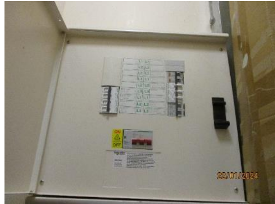
483. Distribution board cleaners room upstairs playgroup
