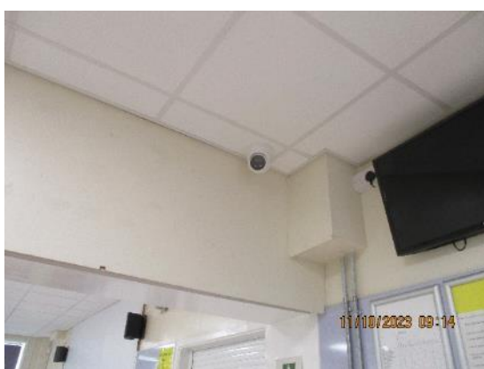
438. CCTV camera – dining room K block
