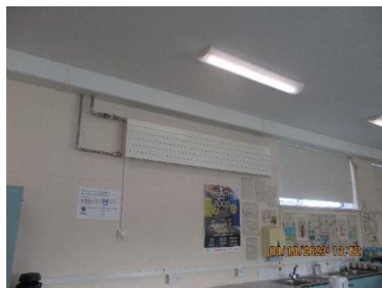
355. High level wall mounted radiator main school.
