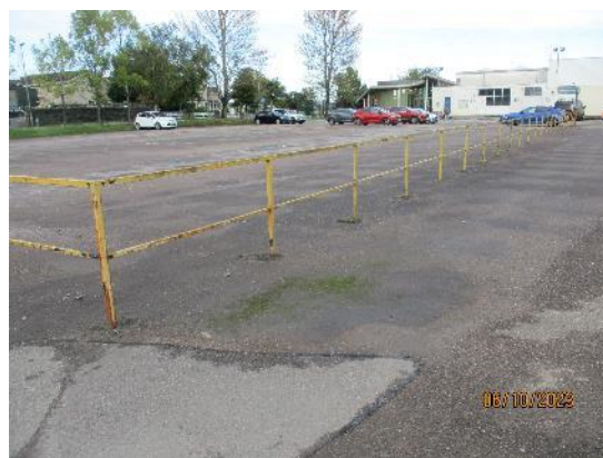
513. Metal bar separation in car park
