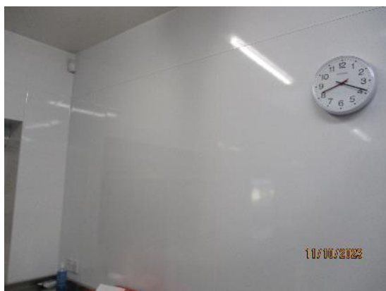
234. Wetwall in Kitchen – Block K
