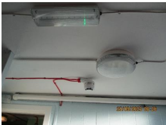
200. Lighting and smoke detection boys toilets.
