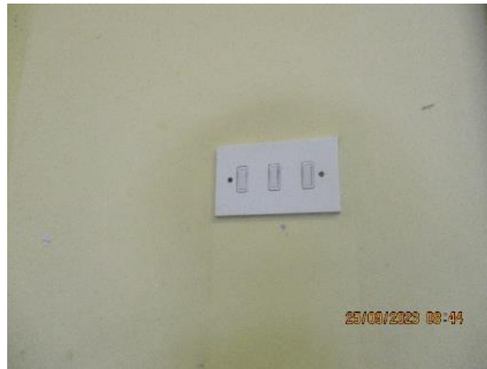
185. Lighting control switch typical.
