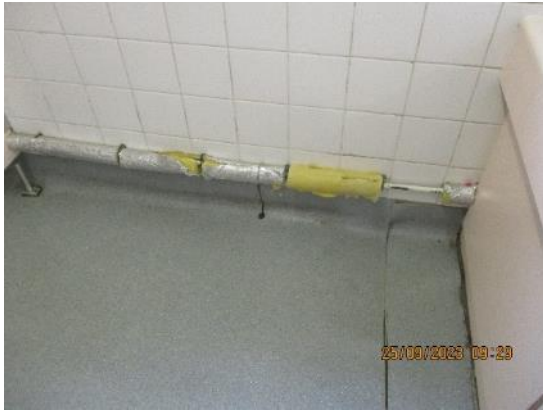
172. Pipework – cold water / girls toilets.
