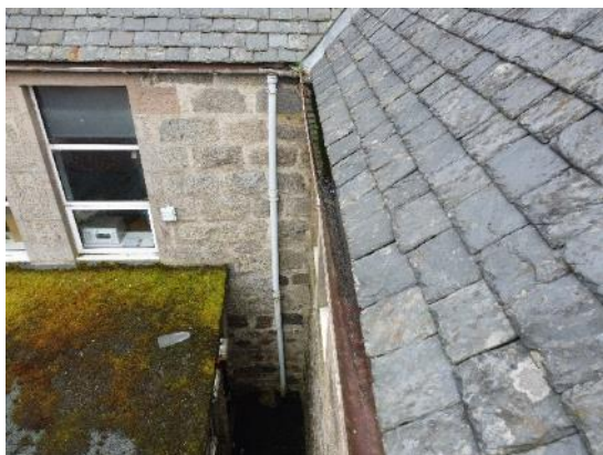
23. Corroded cast iron gutters
