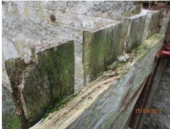
221. Timber rot in frame and slats
