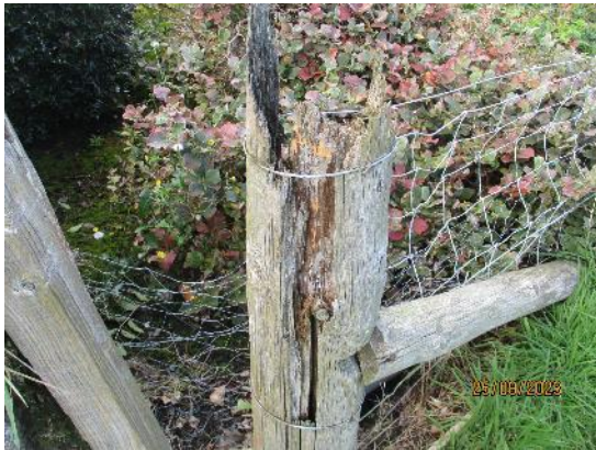
216. Rotten/leaning timber posts
