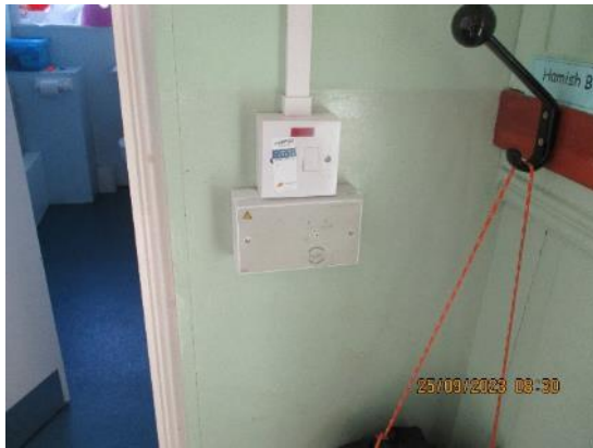
196. Disabled toilet alarm system panel access toilet.
