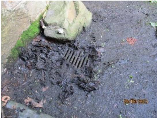
232. Blocked drainage outside Boiler Room
