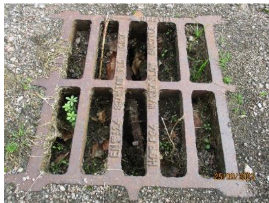
231. Part blocked drainage to playground
