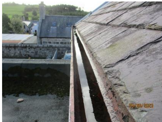
22. Cast iron gutters ponding
