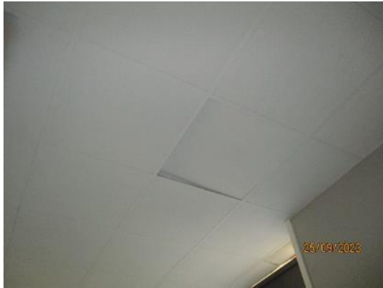
96. Suspended ceiling tiles
