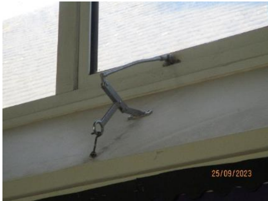
63. High level winding mechanism
