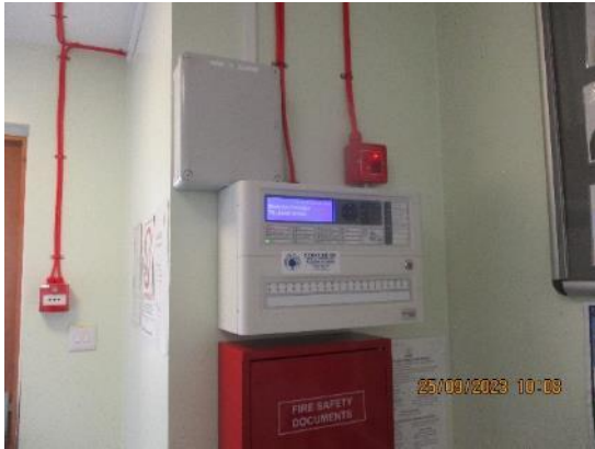
190. Fire alarm control panel and circuit wiring.
