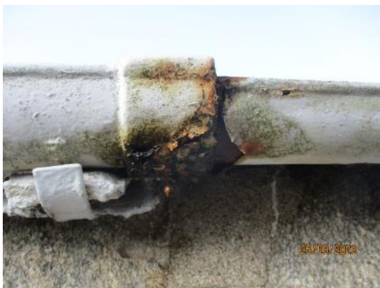
29. Corroded, leaking cast iron gutters
