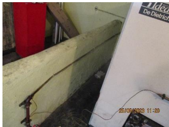
165. Oil supply pipework to boiler.
