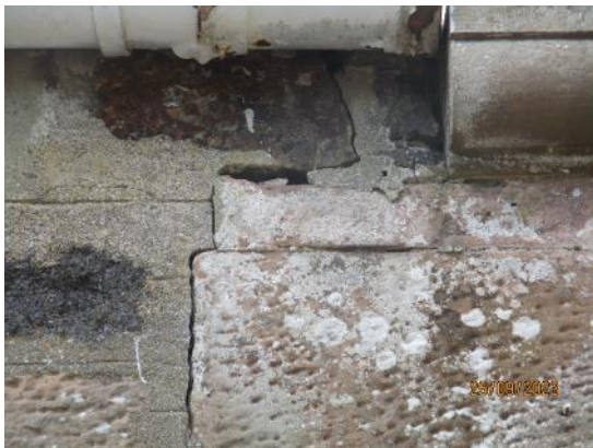
45. Isolated repointing required
