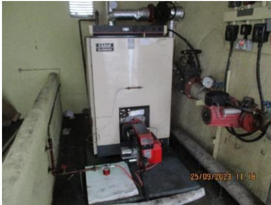
160. Oil boiler – heating system.
