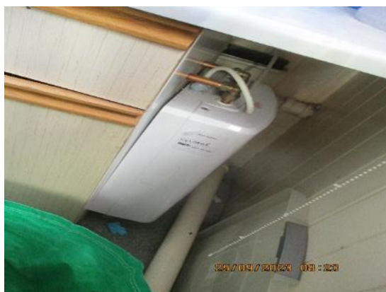
170. Point of use water heater – classroom typical.
