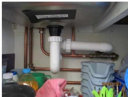
143. UPVC waste pipes
