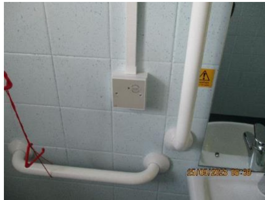
197. Disabled toilet alarm reset unit access toilet.
