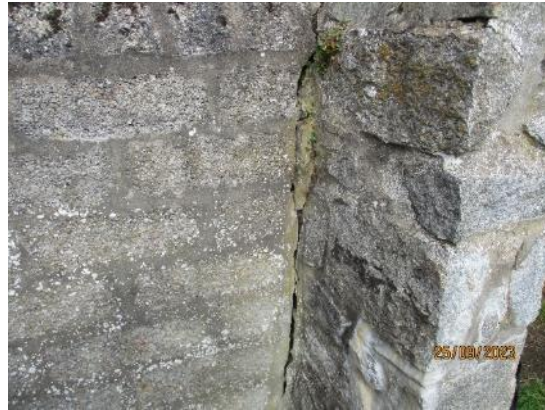
227. Open joint with adjacent block wall
