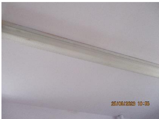
182. Lighting – staff room.
