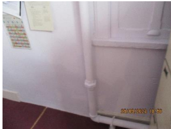
167. Heating system distribution pipework typical.
