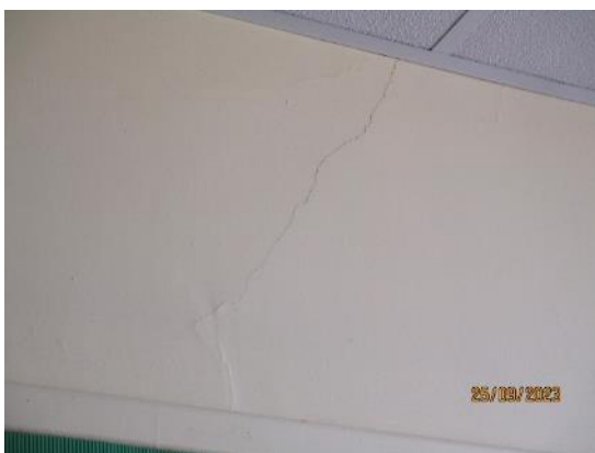
112. Hairline cracking to lath & plaster walls
