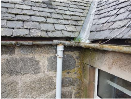
25. Miss-aligned gutters and vegetation
