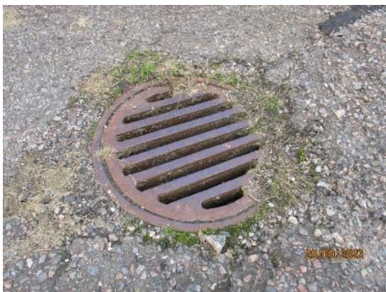
230. Part blocked drainage to car park
