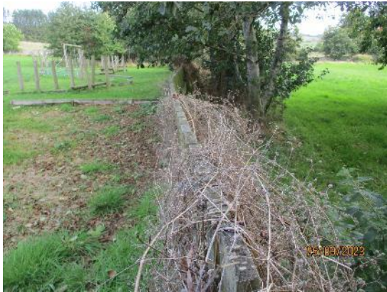
214. Leaning timber boarded fencing
