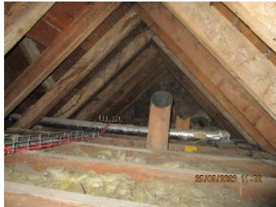
199. Heating pipework in attic space.
