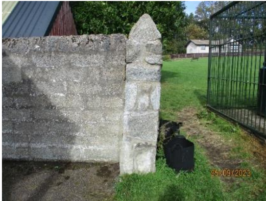
226. Stone wall to sports field - leaning
