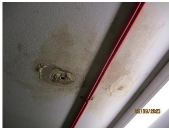
101. Water damaged plasterboard ceilings
