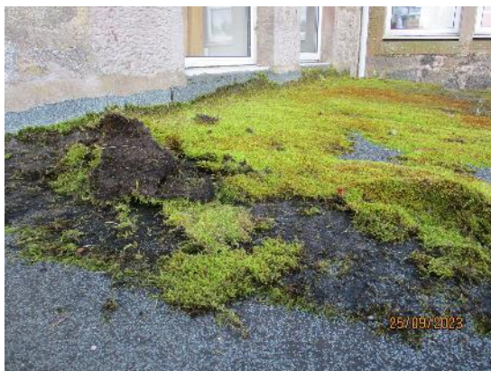
12. Felt roof to Boiler Room has extensive moss growth
