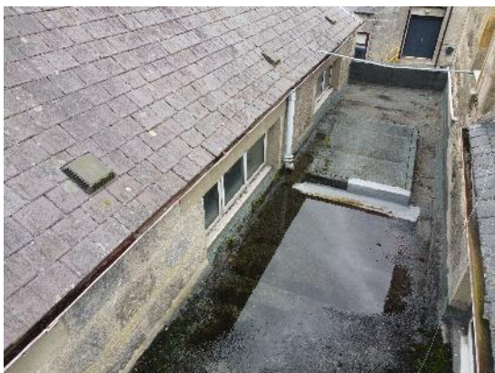
11. Inadequate falls causing ponding
