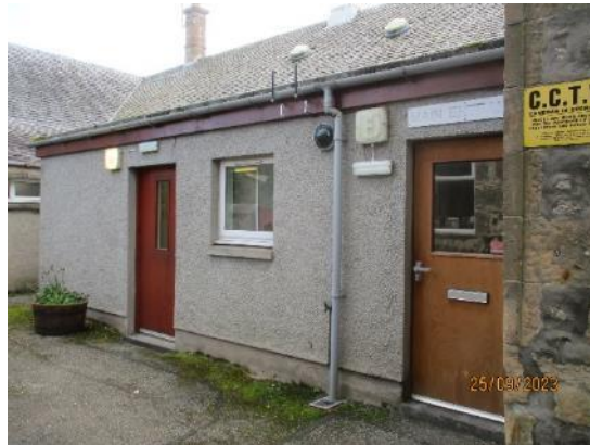
28. UPVC gutter and downpipe
