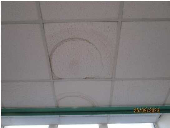
98. Water marked suspended ceiling tiles
