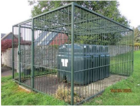
238. Oil tank enclosure
