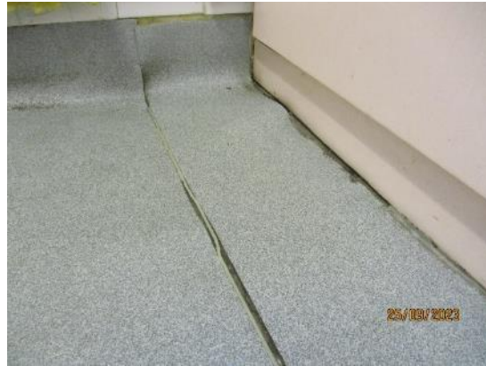
86. Damaged sheet vinyl in Girls toilet
