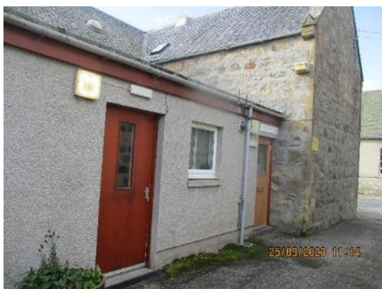
188. External lighting typical.
