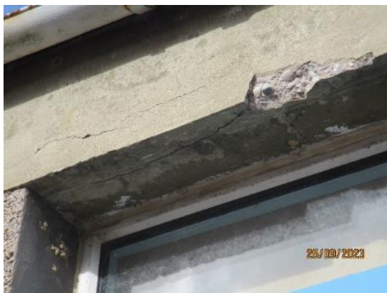
53. Cracked and spalling concrete lintels
