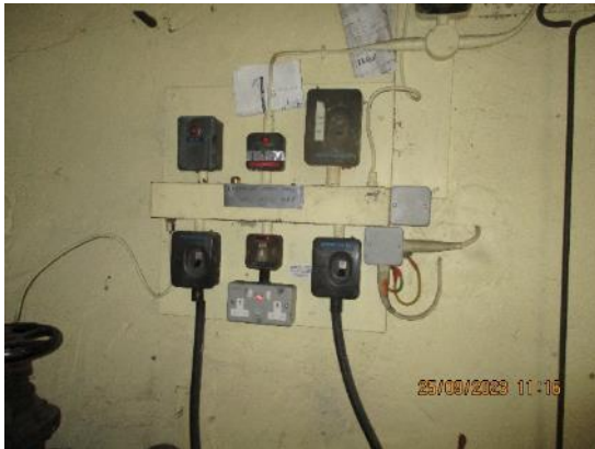
162. Heating system controls – boiler house.
