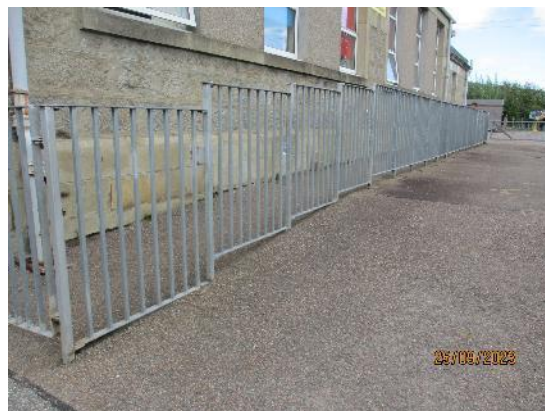
207. Galvanised bar separation fencing
