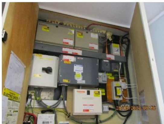
176. Switchgear and distribution boards – reception office cupboard.
