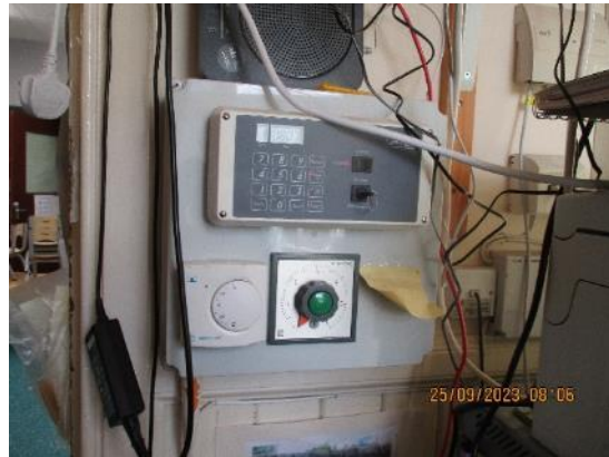
163. Heating programmer – nursery store room.
