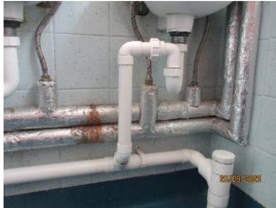
133. UPVC waste pipes
