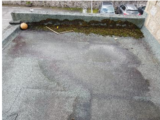
8. Sunken area ponding
