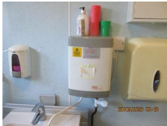
169. Point of use water heater. Access toilet.
