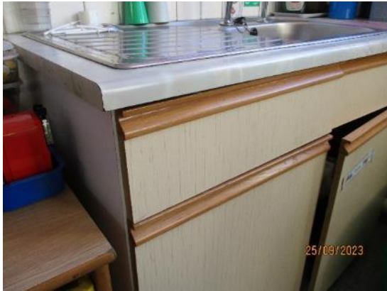
156. Damage to doors and drawers
