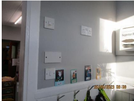
179. Sockets and switches typical.
