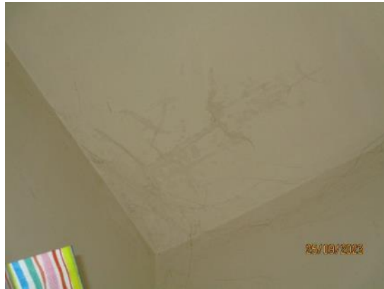
105. Hairline cracking to lath & plaster ceilings
