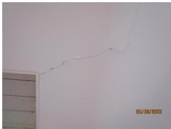
107. Hairline cracking at loft hatch
