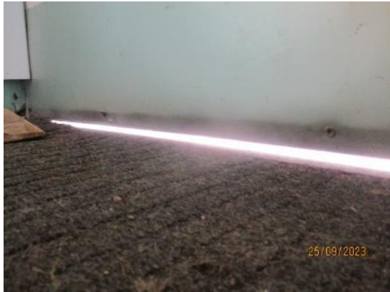
55. Daylight visible around external doors
