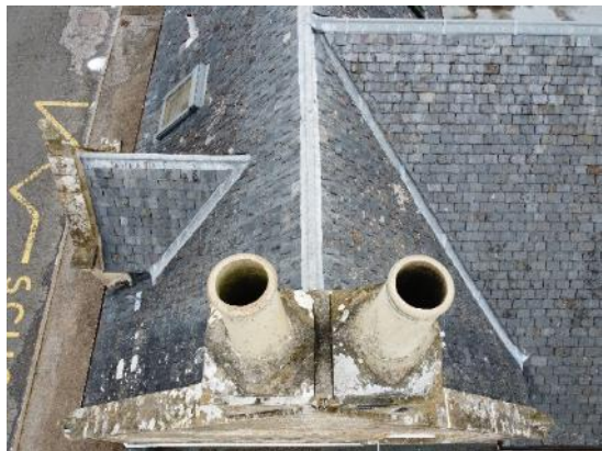
36. Open, uncapped chimney pots
