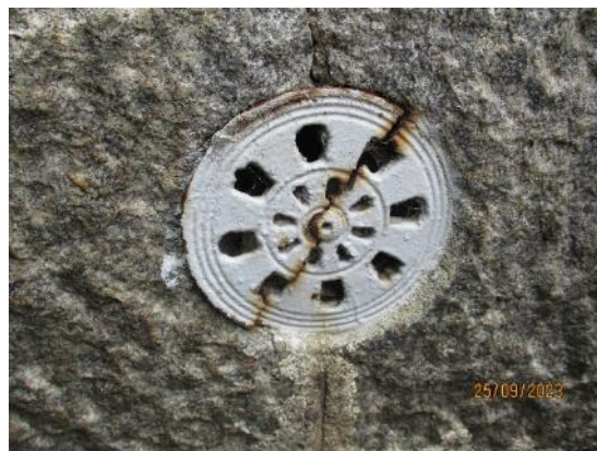
42. Broken vent covers
