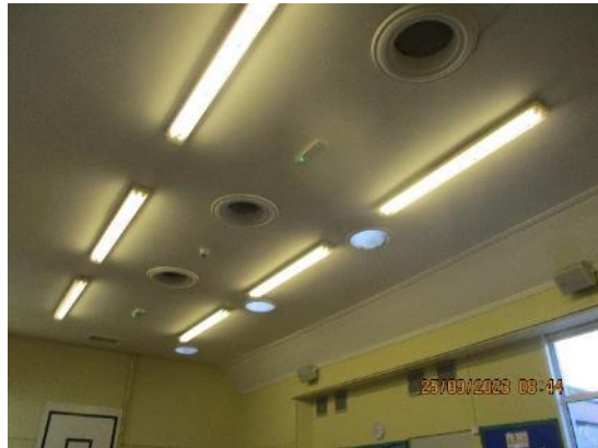
181. Lighting – GP hall.
