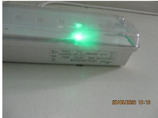
187. Emergency lighting internal typical LED.
