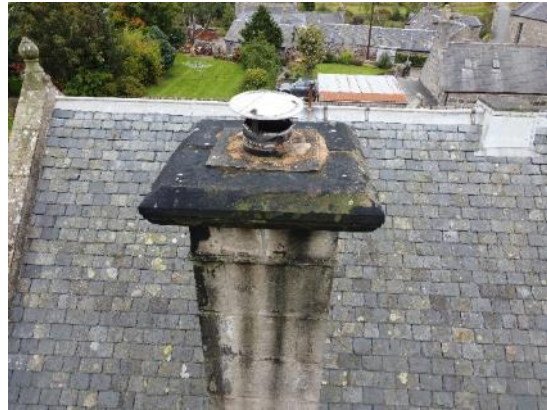
161. Oil boiler flue termination
