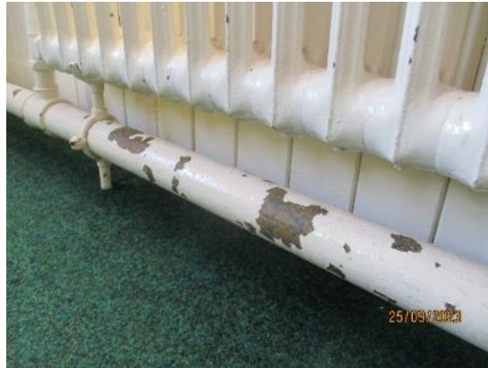
151. Metal heating equipment
