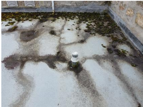
15. GRP roof blistering and crazing
