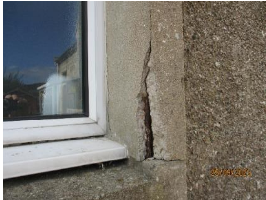
52. Exposed reinforcement to window surrounds
