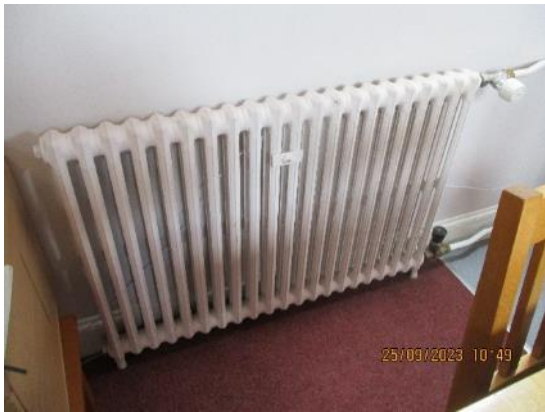
166. Cast iron section radiator staff room 2-23
