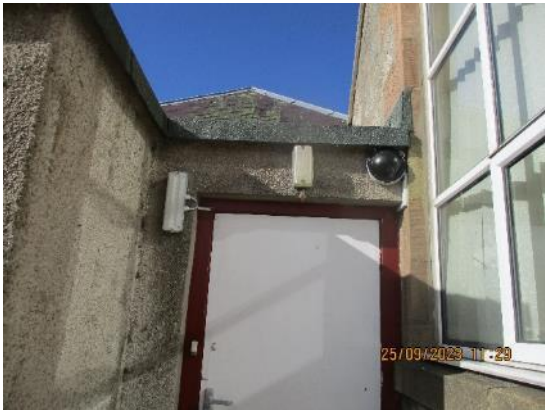
198. CCTV camera – south external entrance door.
