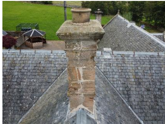
34. Eroded stone chimney stack
