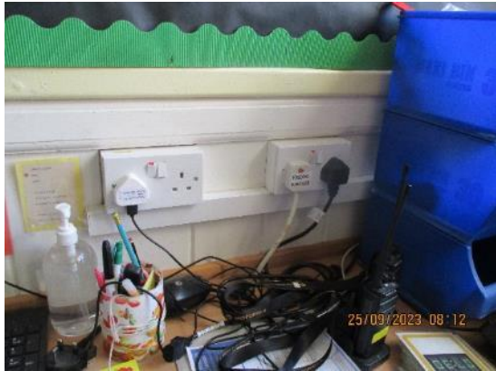
178. Sockets and plastic trunking typical.
