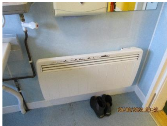
201. Electric convector – access toilet.
