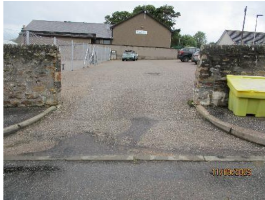
155. Eroded car park entrance
