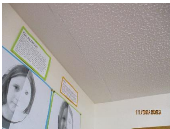
73. Hairline cracks at board edges
