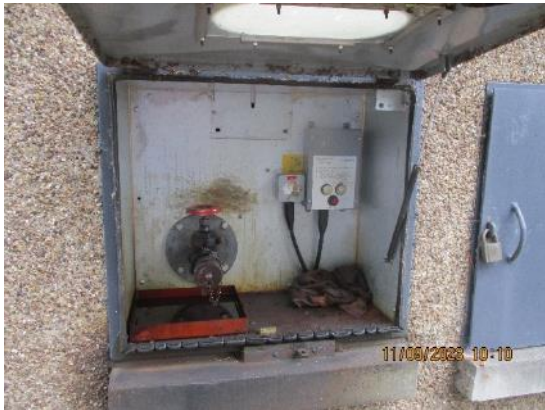
120. Oil tank filling point and fill alarm system. 1/20
