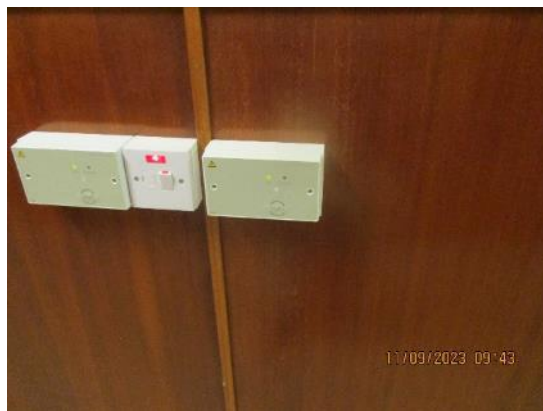
147. Disabled toilet alarm systems 1/7 and 1/6 toilets.
