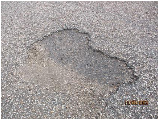
156. Potholed car park
