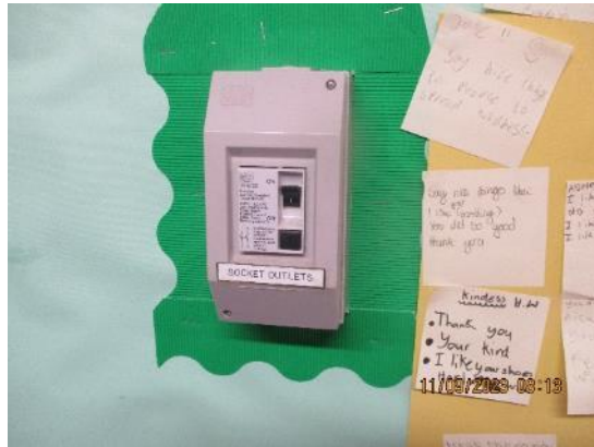
133. Classroom socket RCD unit. 1/13
