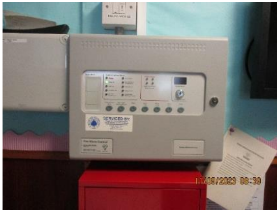
142. Fire alarm call point.
