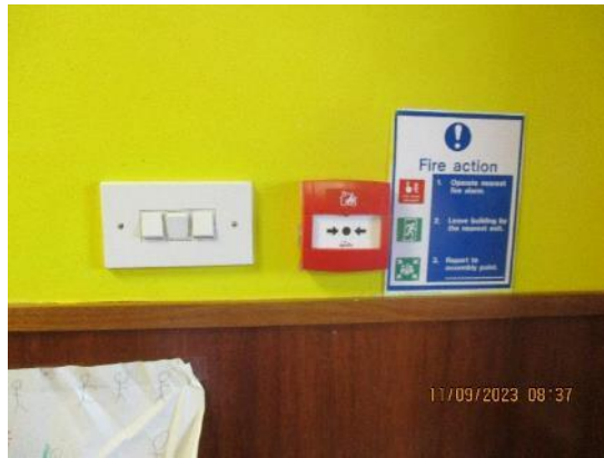
143. Fire alarm call point typical.
