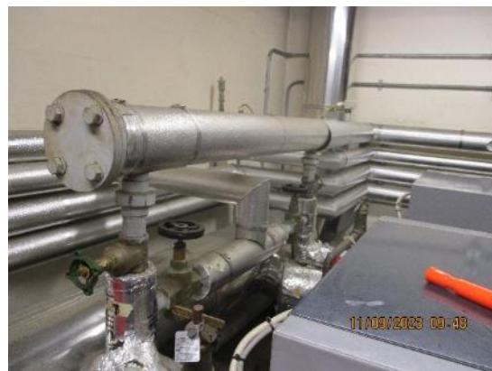
117. Heating pipework in boiler house 1/19.
