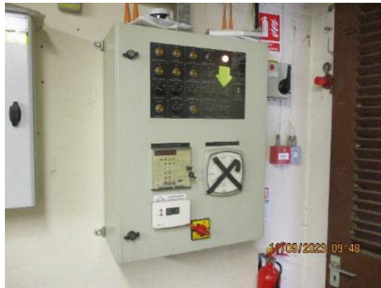
113. Heating system control panel. 1/19
