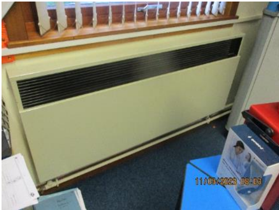
114. Convector heater typical.
