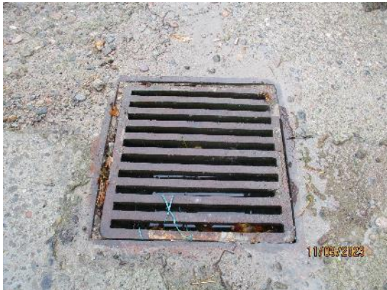
192. Surface water pot gullies
