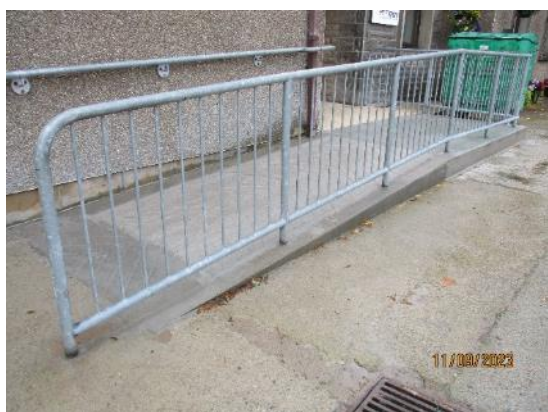
55. Galvanised tubular guardrail
