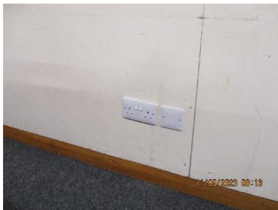
134. Flush fitted wiring accessories typical.
