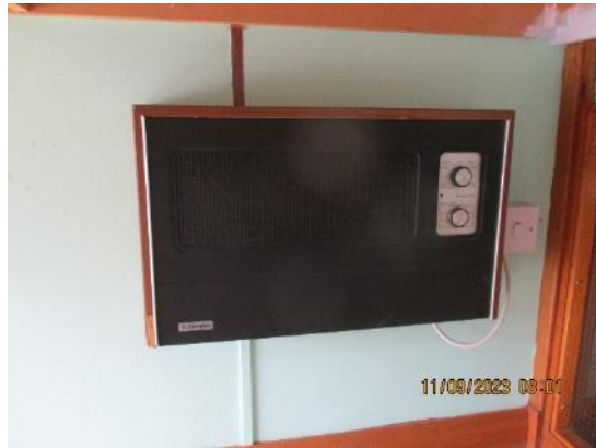
115. Electric convector heater. 1/1 entrance lobby.
