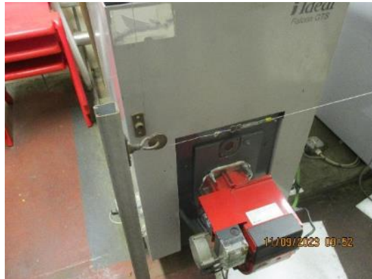
145. Fire wire – oil shut off system 1/19.
