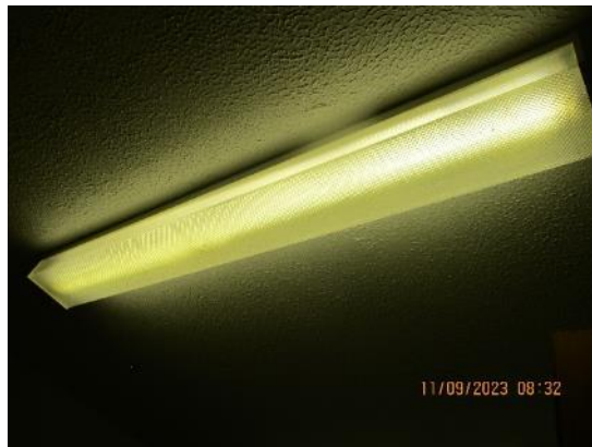
139. Lighting girls toilets 1/15.
