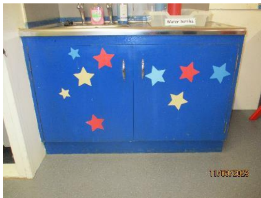
107. Timber sink base units
