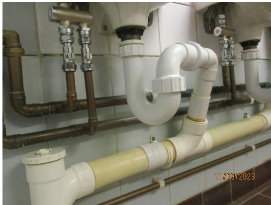
93. PVC waste pipes
