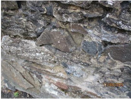
184. Stone walls require isolated repointing
