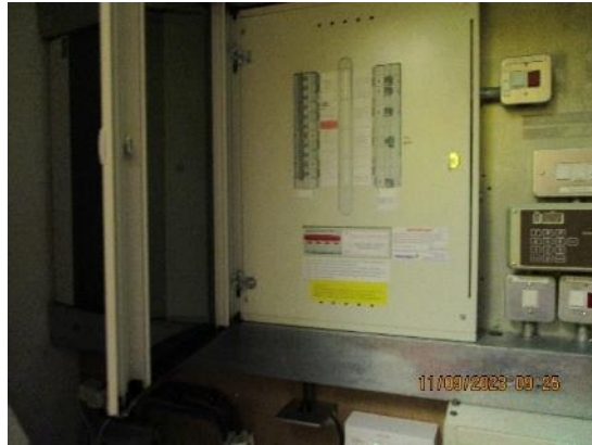
131. Distribution board L+P 2- 1/5 cupboard.
