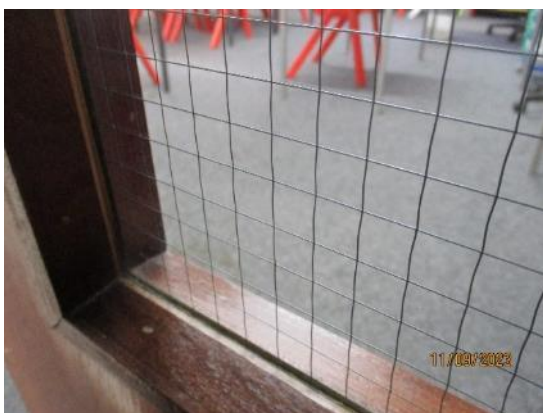
85. Georgian wired glazing
