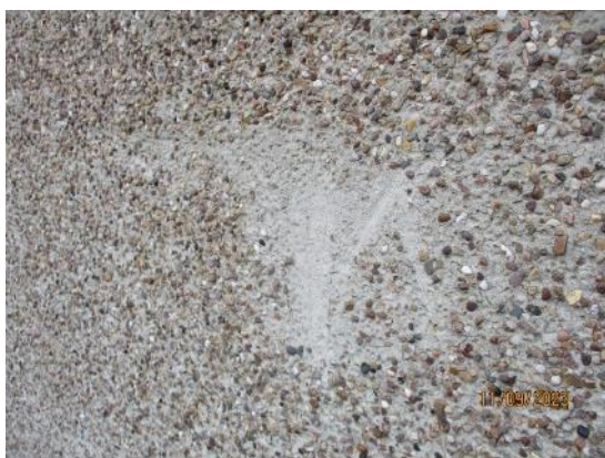
36. Eroded roughcast surface
