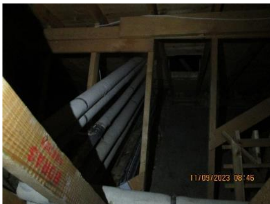
116. Heating pipework – attic space.
