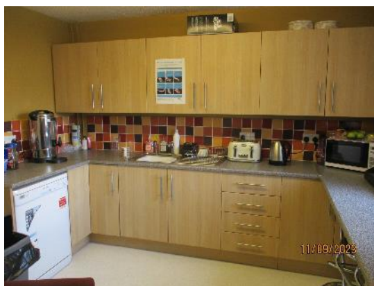
109. Staff room base and wall units
