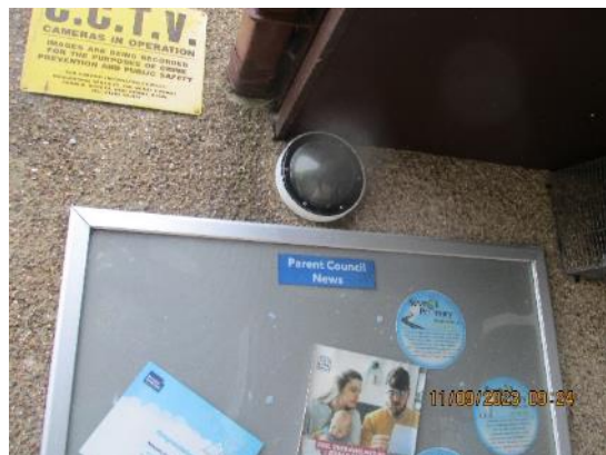
150. CCTV camera main entrance.
