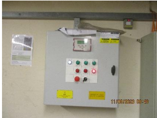
119. Biomass loop control panel 1/19.
