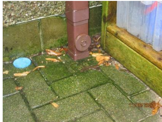
22. Downpipes blocked and leaking
