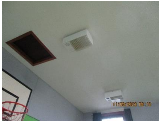
137. Lighting – main hall 1/18.
