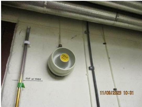
144. Fire alarm bell – typical. Boiler house 1/19.
