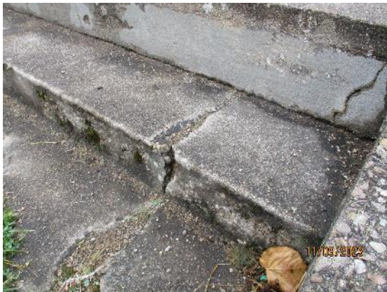
172. Cracked concrete steps
