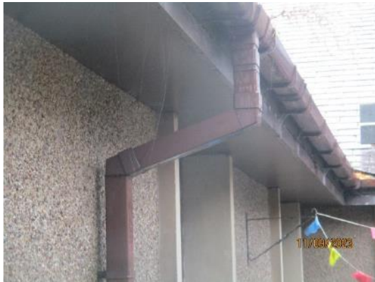
21. UPVC rainwater downpipes
