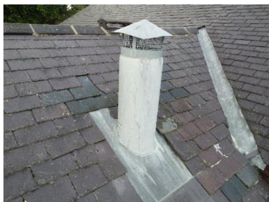
153. Kitchen extract ductwork termination.
