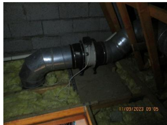
129. Extract fan and ductwork from kitchen canopy in attic space.
