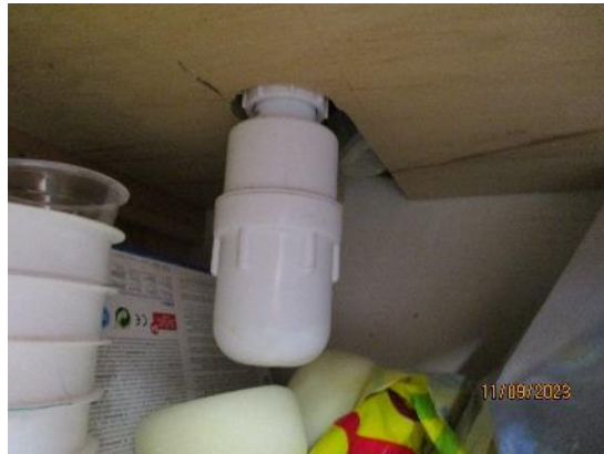
102. PVC waste pipes
