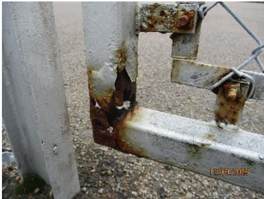
180. Corrosion to metal frame
