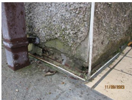
35. Damaged roughcast finish
