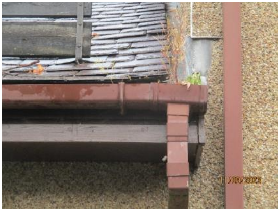
27. Vegetation in gutters
