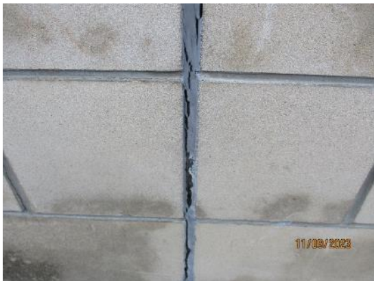
33. Expansion joints require resealing
