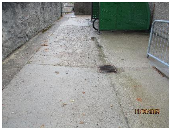
165. Eroded concrete to front entrance
