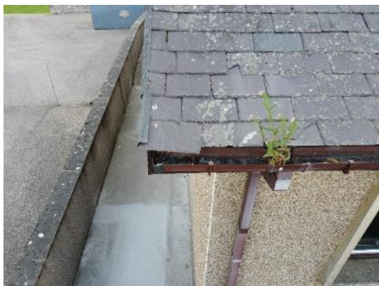
5. Slipped and broken slates
