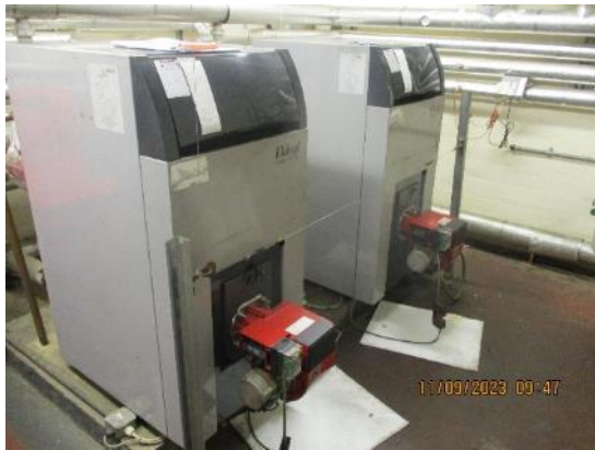
112. Oil fired boilers. 1/19
