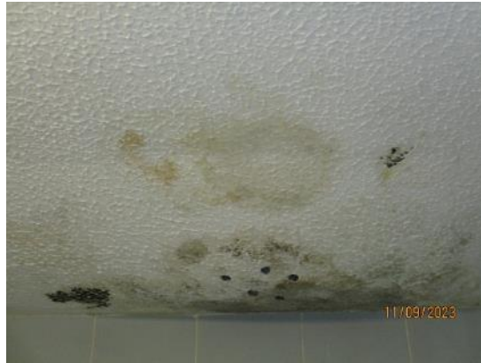
70. Water penetration and damage
