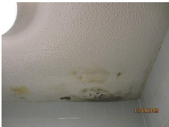
103. Water damaged plasterboard ceilings
