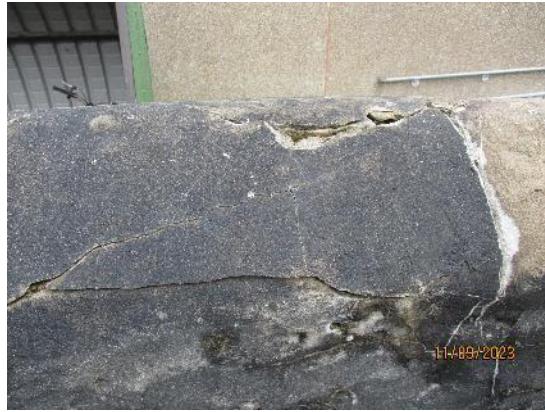
185. Cracked render coping
