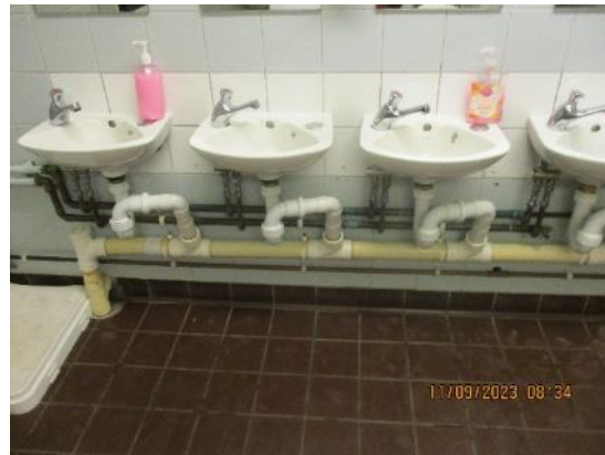
125. Cold water pipework girls toilets 1-15.
