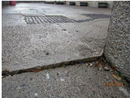
163. Raised edges and trip hazards
