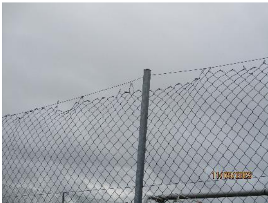
174. Isolated areas of damage
