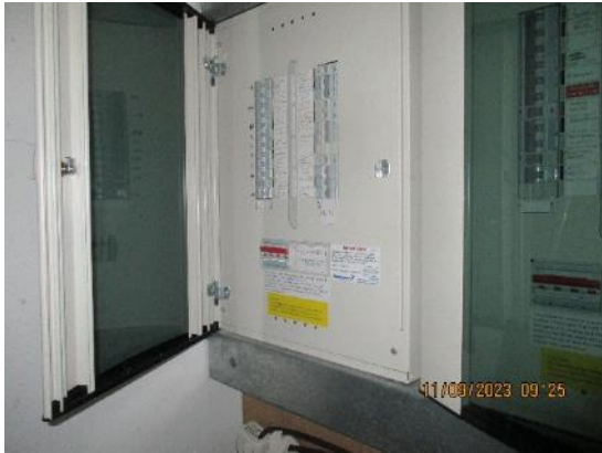
130. Distribution board L+P 1. – 1/5 cupboard.
