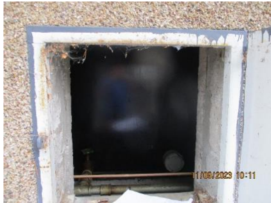
121. Oil tank in bunded room. 1/20.
