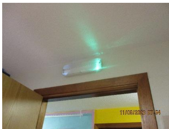
141. Emergency lighting office 1/3.
