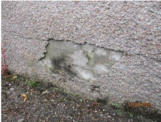
190. Spalling roughcast surface
