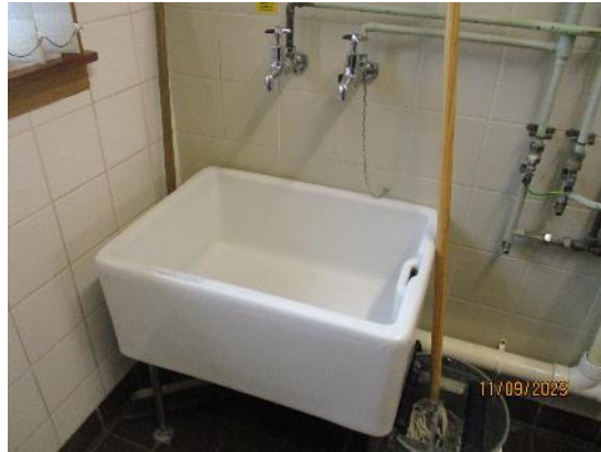
100. Butler cleaners sinks
