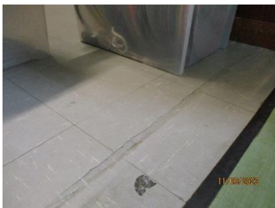
62. Vinyl tiles cracked and breaking up
