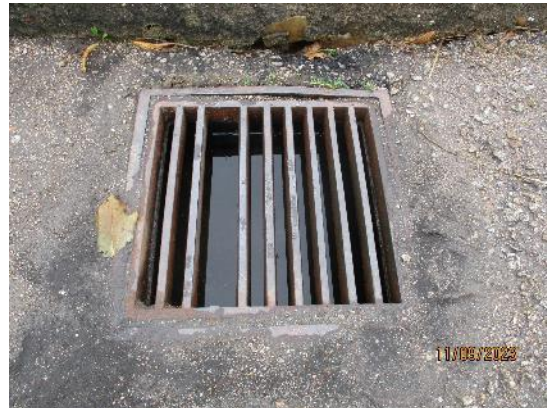
193. Isolated damage to gully gratings
