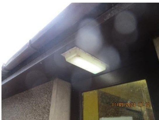
140. External maintained emergency light.
