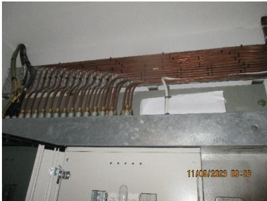
132. General wiring exiting DB L+P1. 1/5 cupboard.
