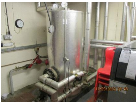
122. Hot water calorifier 1/19.
