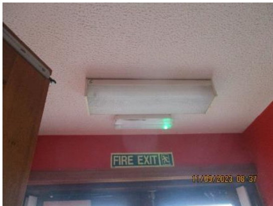
138. Lighting boys toilets 1/16.
