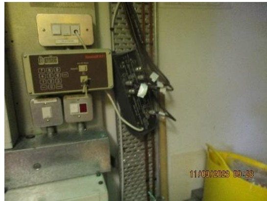
149. TV aerial amplifier unit – 1/5 cupboard.
