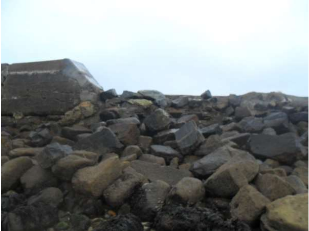
Displaced rock armour and wall section at root of West Pier
