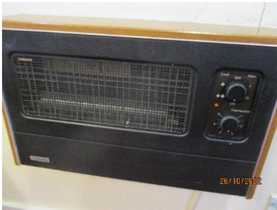
99. Electric fan convector classroom typical
