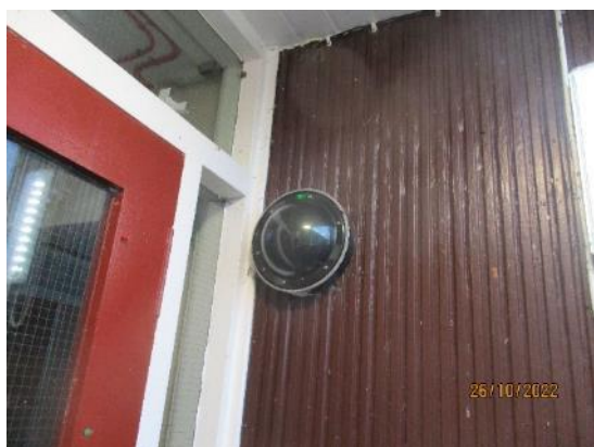
135. CCTV Camera – Main reception
