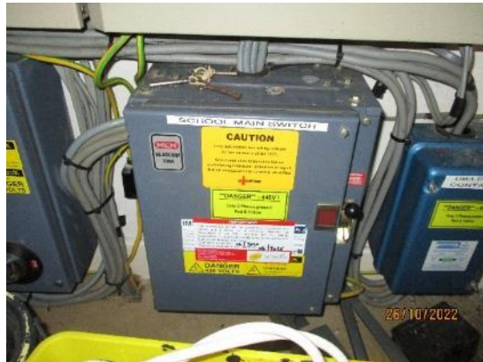
114. Switchgear – main school isolator.
