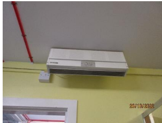
100. Electric fan heater toilet and kitchen typical
