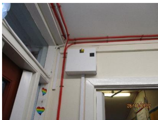
132. Fire alarm interface at main entrance security door
