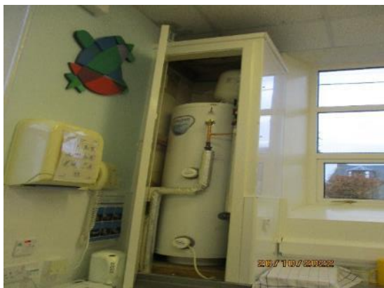
103. Hot water tank – kitchen old block
