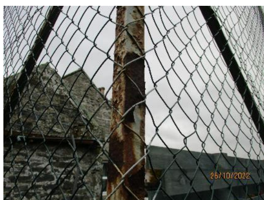
54. Corroded fence posts
