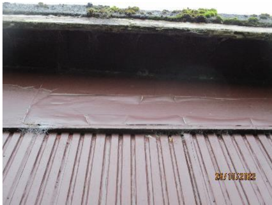
49. Timber cladding flaking and peeling
