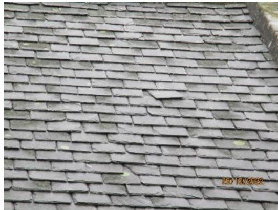
4. Isolated slipped and missing slates
