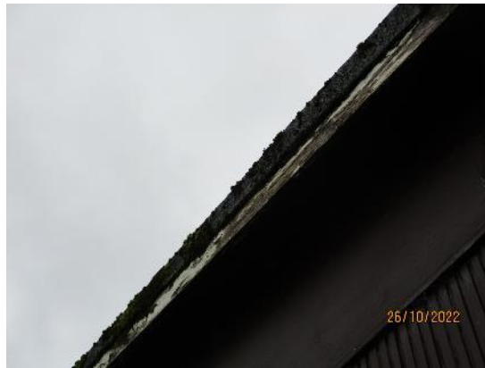
50. Timber fascia boards peeling
