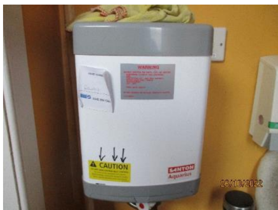
105. Point of use water heater old block toilet
