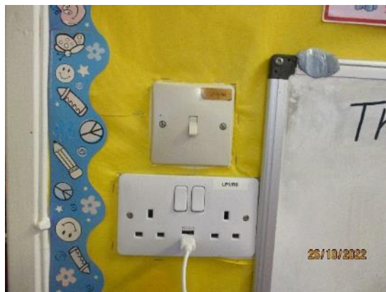
116. Switches and sockets typical.
