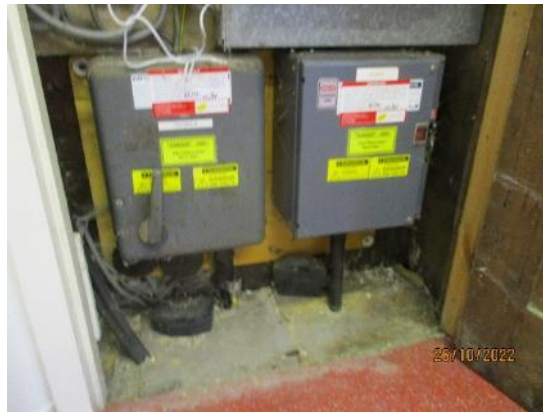
118. Switchgear – main switches old building.
