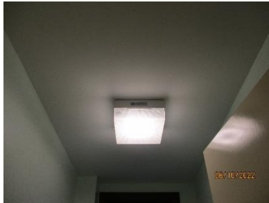
120. Lighting staff toilet
