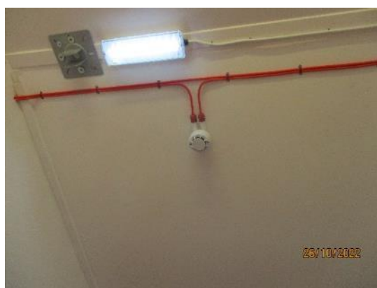
130. Fire detector head and wiring class block typical
