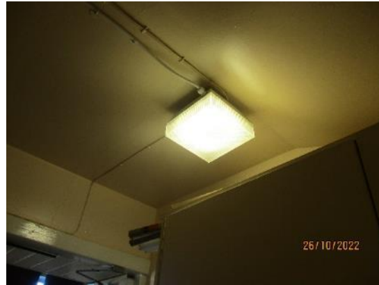
124. Lighting – store typical.
