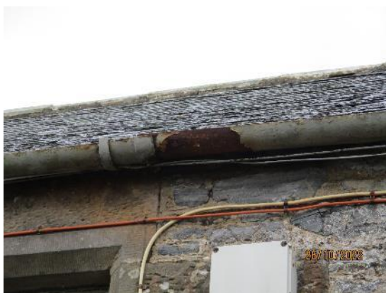
53. Cast iron peeling
