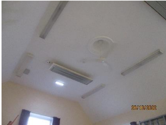
111. Destratification fans – assembly hall.
