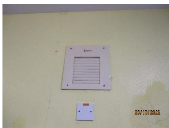
109. Extract fan – boys toilets class block
