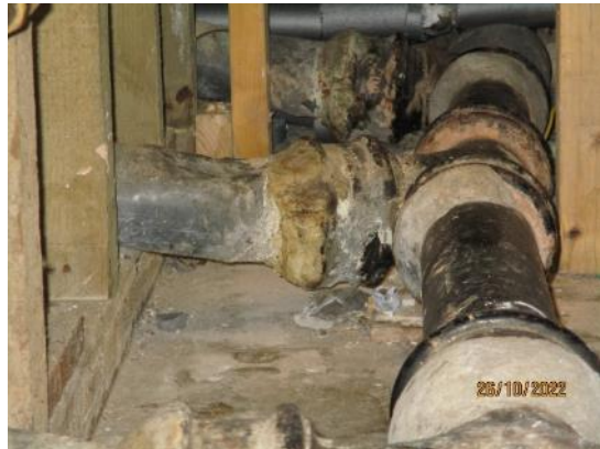
90. Damaged lead waste pipes
