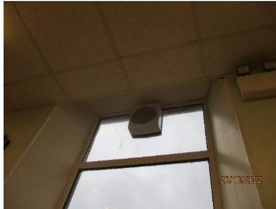
112. Extract fan. Old block kitchen.
