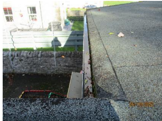
16. Poor fall and standing water
