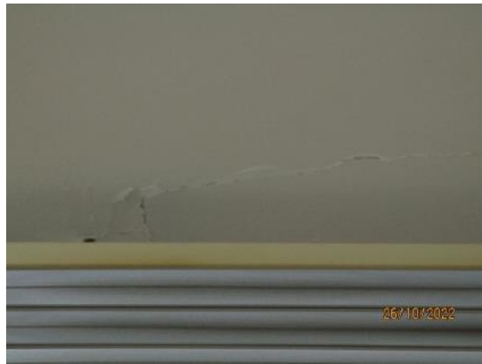
72. Lath and plaster - cracked
