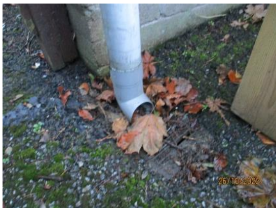
23. UPVC rainwater downpipes
