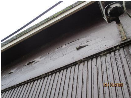
51. Timber cladding flaking and peeling
