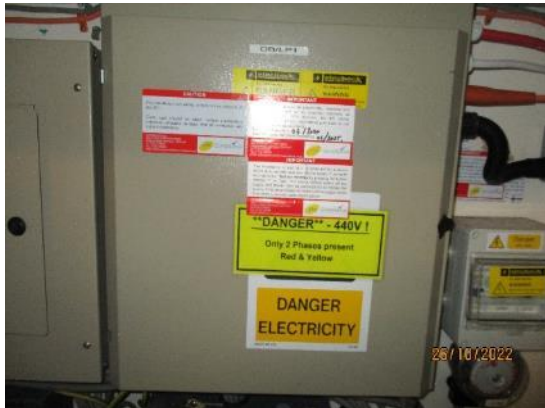
113. Distribution board – power and lighting. Class block
