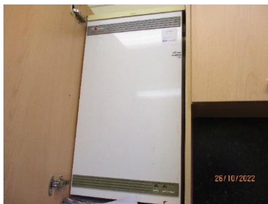
106. Point of use water heater. Staff room class block.
