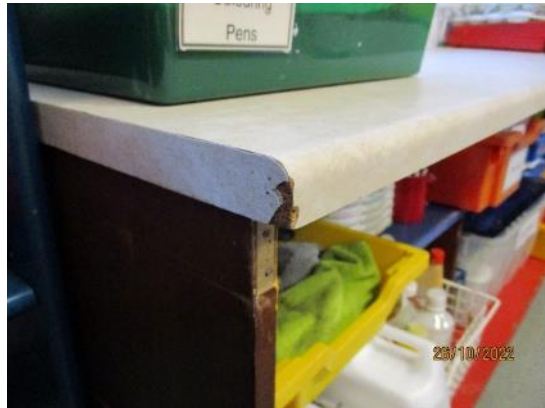
96. Damage to worktops
