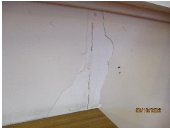
79. Surface damage to plasterboard
