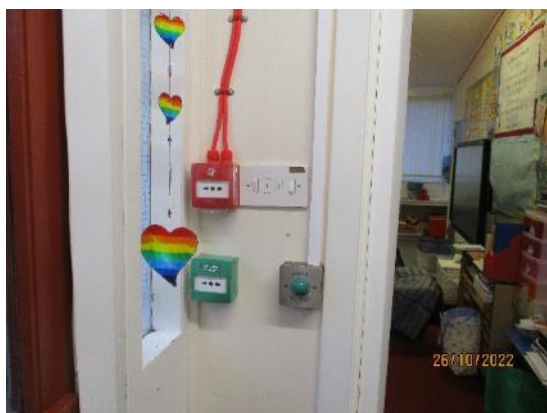
139. Security door release devices. Main entrance
