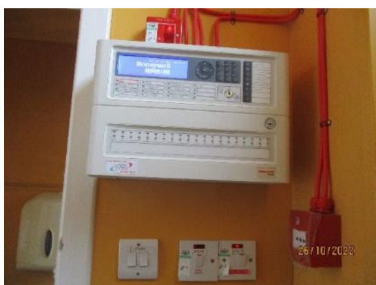
133. Fire alarm panel old building
