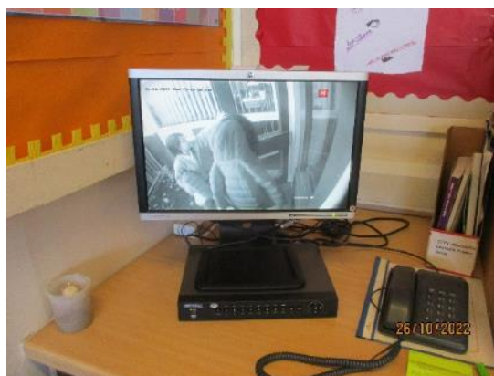
136. CCTV monitor and processor classroom 2
