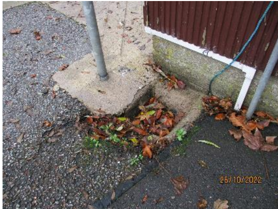
153. Blocked surface water drainage
