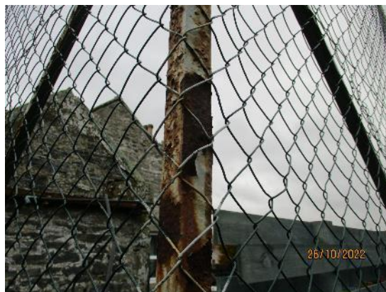
146. Corrosion of steel posts
