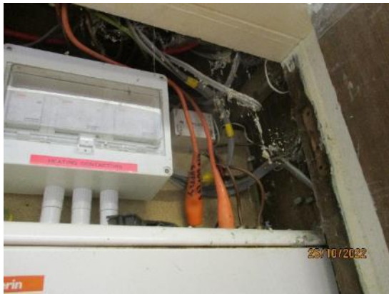
117. General wiring – old building switchgear cupboard.
