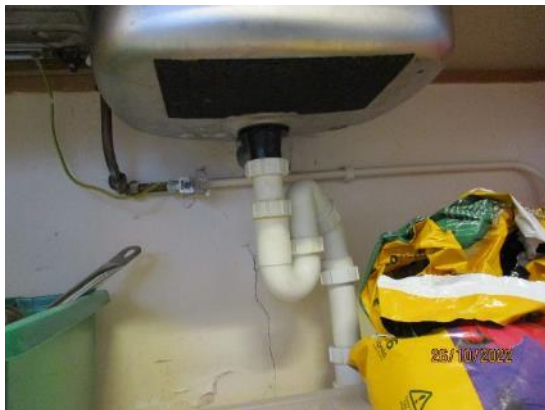
85. UPVC waste pipes
