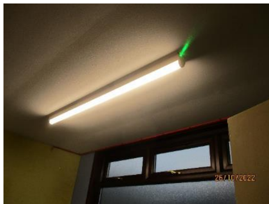
122. Lighting boys toilet class block.
