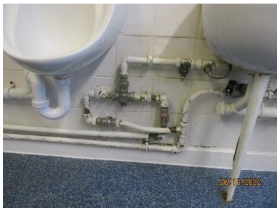
107. Hot and cold water pipework – boys toilets class block
