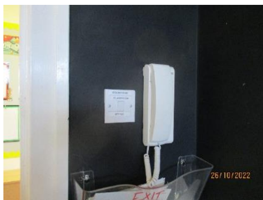
138. Security door release handset classroom 2
