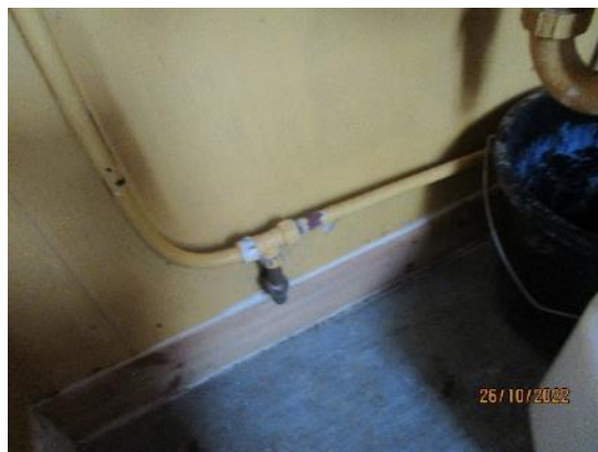
108. Cold water pipework – old building toilet.
