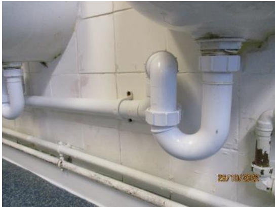
89. UPVC waste pipes
