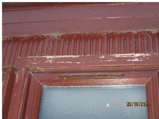
52. Window surrounds peeling
