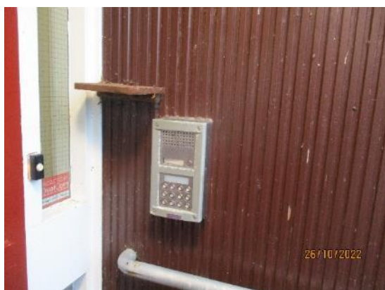
137. Door security intercom – main entrance
