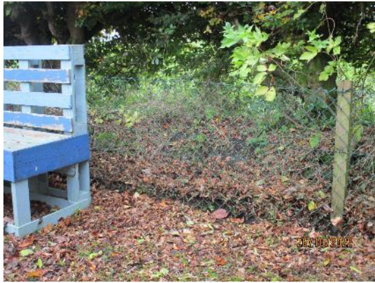
147. Low level chainlink fencing
