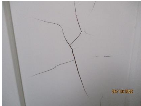
91. Cracked paint to doors
