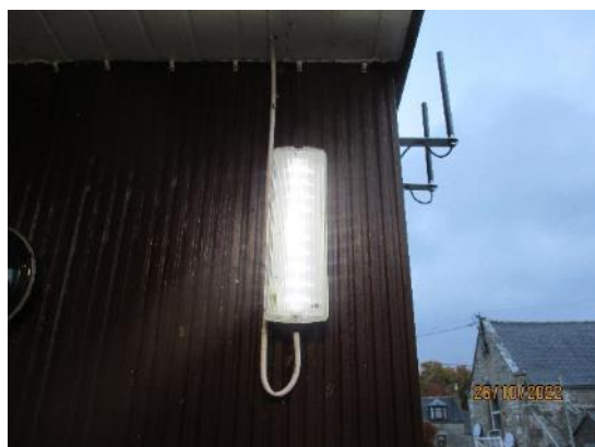
128. External emergency light class block.
