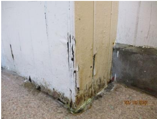
84. Timber decay in linings
