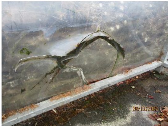
155. Damaged PVC cladding
