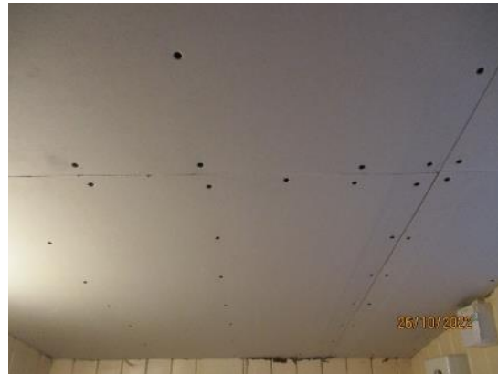
74. Plasterboard (not taped & filled)
