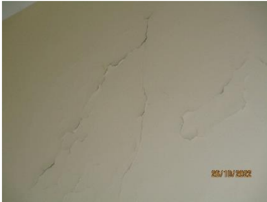
82. Cracked lath & plaster walls
