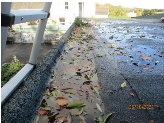
17. Felt box gutters blocked
