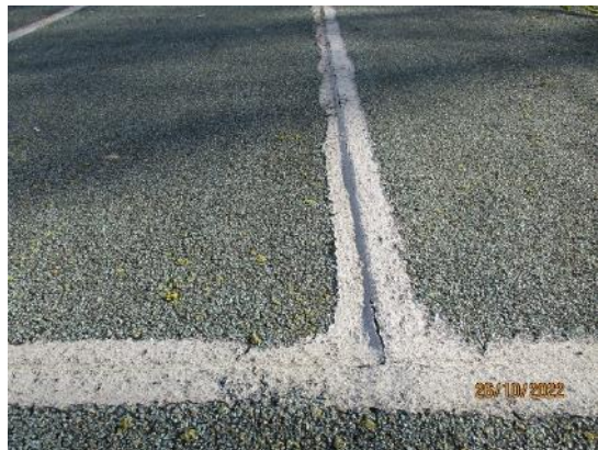
10. Previous joint repairs are failing
