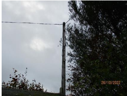
160. BT utility pole
