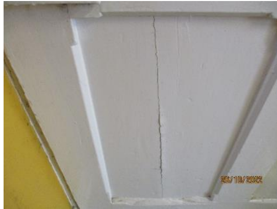
89. Damage to timber doors
