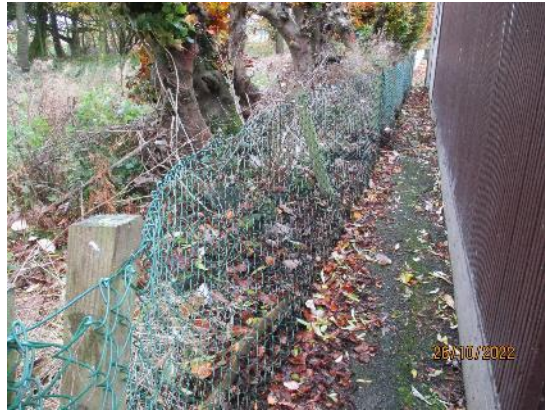
148. Rotten timber posts, damaged chainlink
