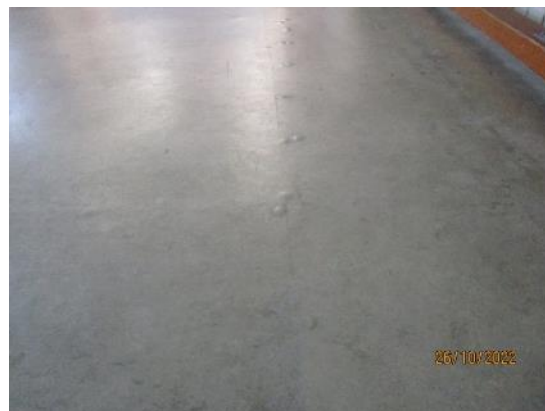
59. Uneven timber suspended floor – Old building
