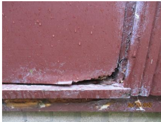
38. Timber decay in doors
