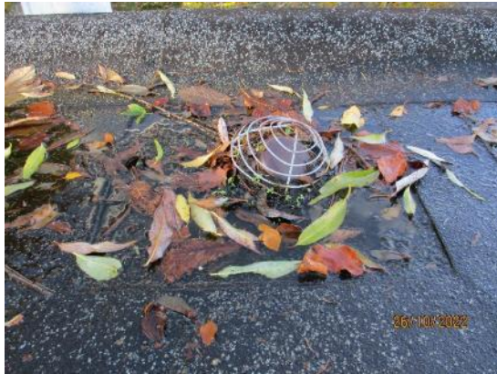
19. Blocked rainwater outlets
