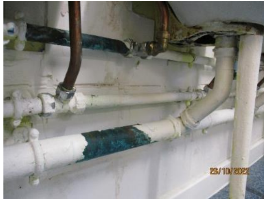
88. Copper waste pipes
