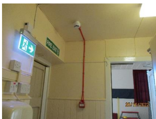
134. Fire alarm devices and wiring old building typical
