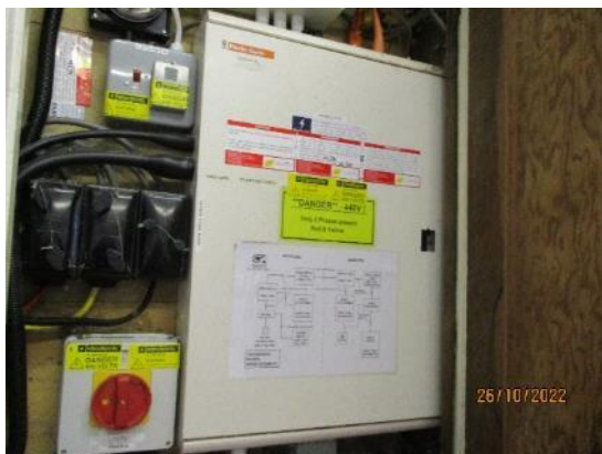
115. Distribution board – lighting and power old building
