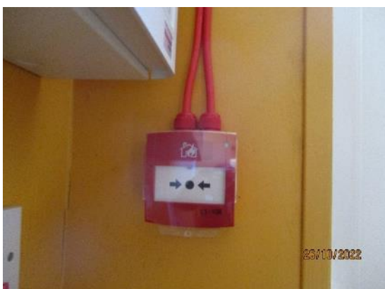
131. Fire alarm system call point typical
