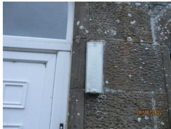
126. External emergency light old building.
